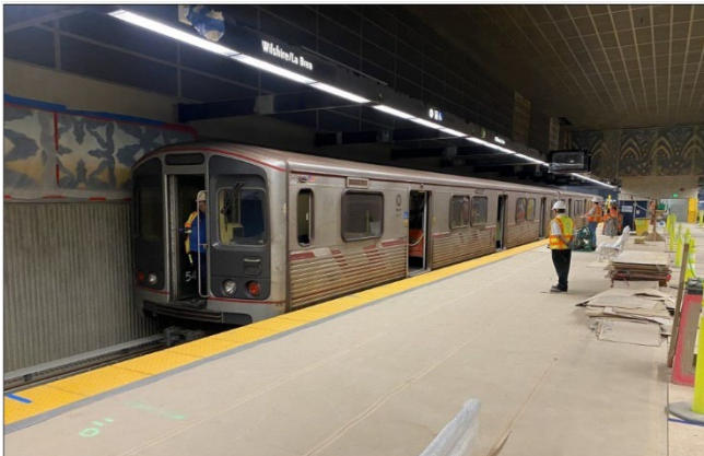
Wilshire/La Brea Station Dead Car Train Clearance Test
