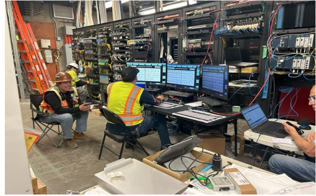
Wilshire/La Brea Station Emergency Management Panel (EMP) Acceptance Test
