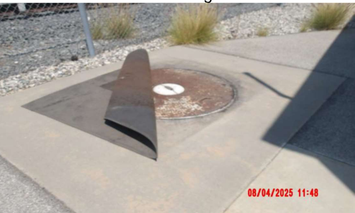
Diesel fuel vault tank TPSS generator enclosure.
