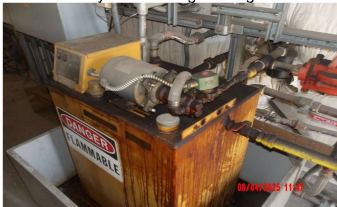
Diesel fuel day tank existing TPSS generator
