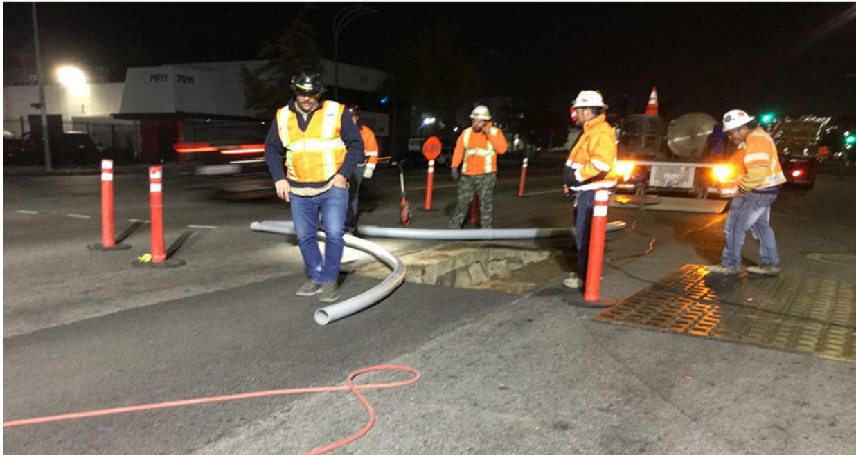
WA Rasic removed road plates at proposed connection points at Northbound lanes of Van Nuys Blvd.
