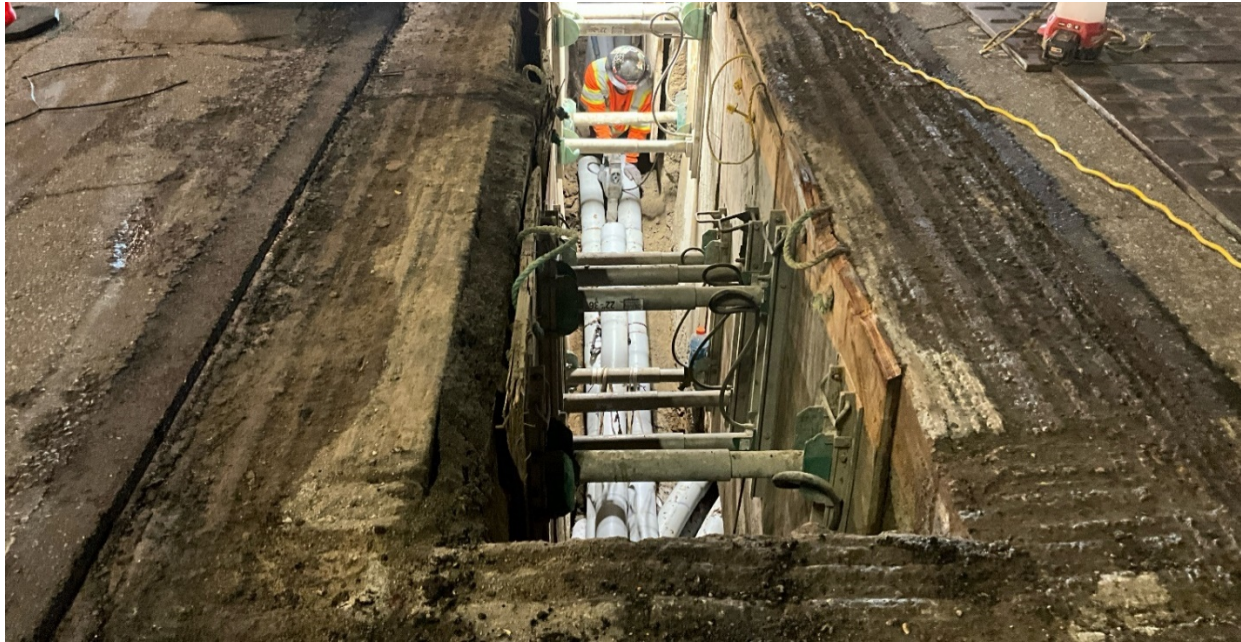
WA Rasic connecting to existing duct bank. Installed (6) 5" conduits to side of trench and (3) 5" conduits straight. Location: Northbound lanes of Van Nuys Blvd. at intersection of Vanowen St.
