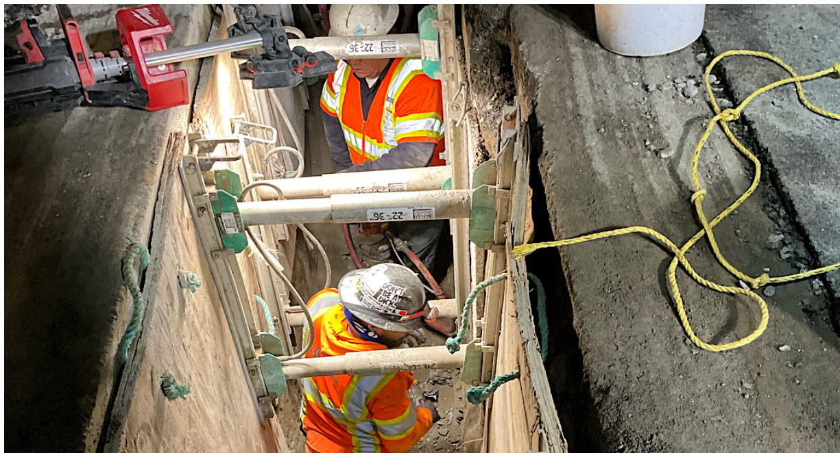
WA Rasic removing concrete encasement to connect to previously installed conduits at mainline A. Location: Northbound lanes of Van Nuys Blvd. at intersection of Vanowen St.
