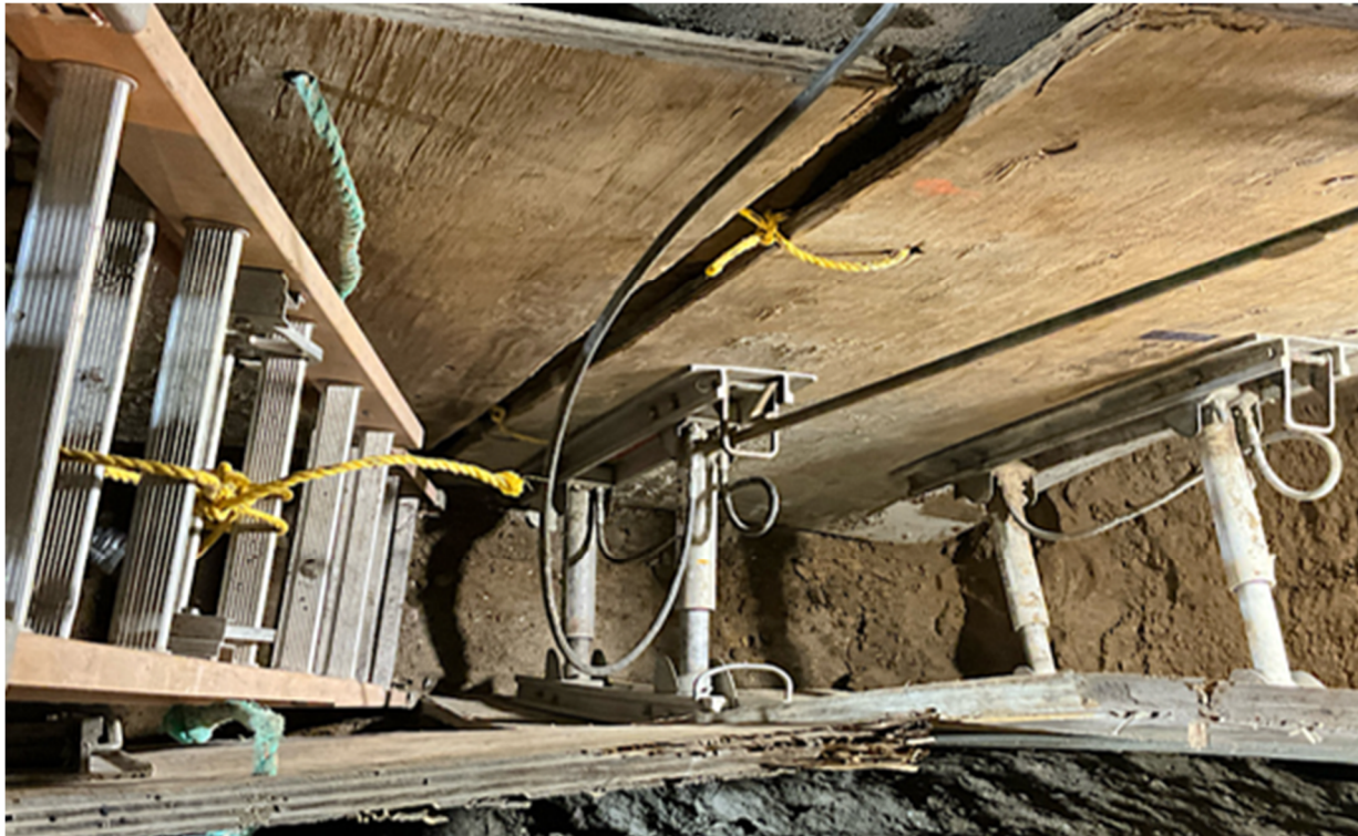
WA Rasic excavated to locate 18" storm drain. Location: Northbound lanes of Van Nuys Blvd. at intersection of Vanowen St.
