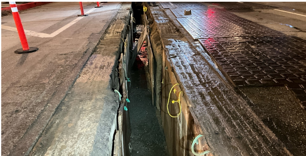
WA Rasic removed shoring after encasement was complete Bulkhead at south end. Location: Northbound lanes of Van Nuys Blvd. at intersection of Vanowen St.
