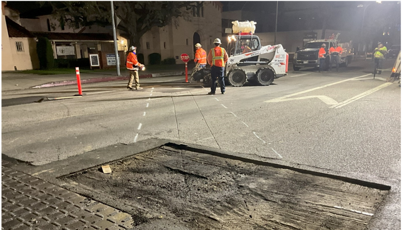
WA Rasic laid out for trench, grind and ground asphalt to recess road plates. Location: Northbound and Southbound lanes of Van Nuys Blvd. at intersection of Hart St.
