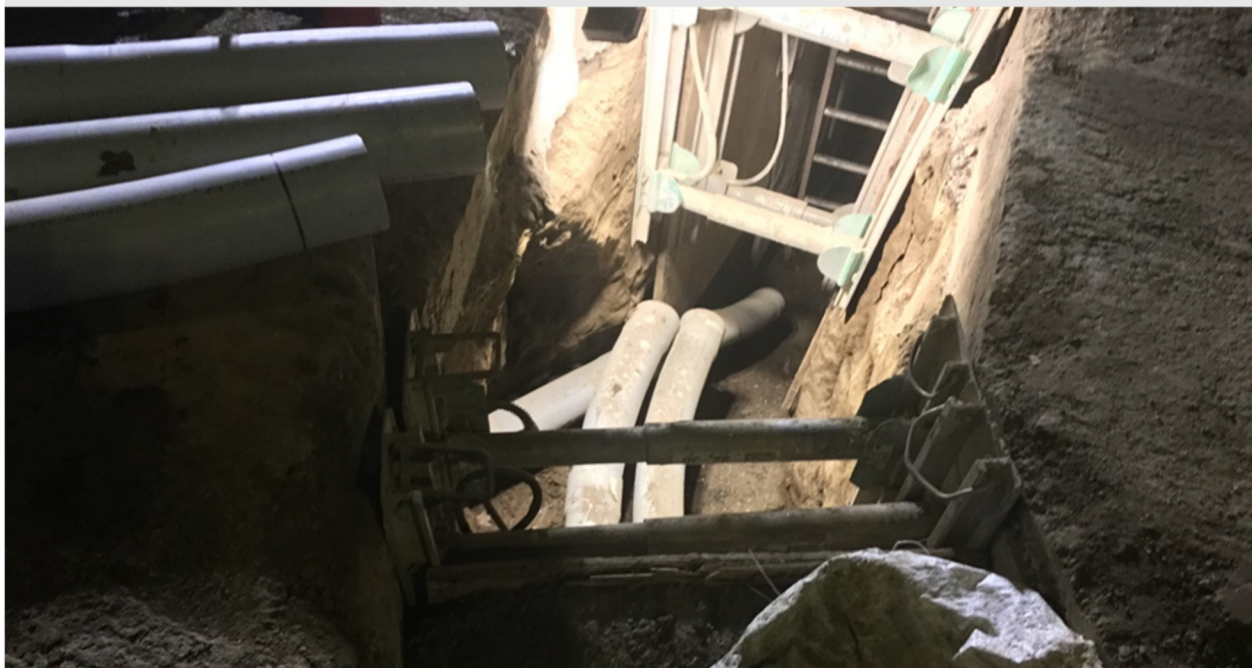
WA Rasic excavating and installing conduits 31, 32, 33 and 21. Location: Northbound and Southbound lanes of Van Nuys Blvd. at intersection of Hart St.
