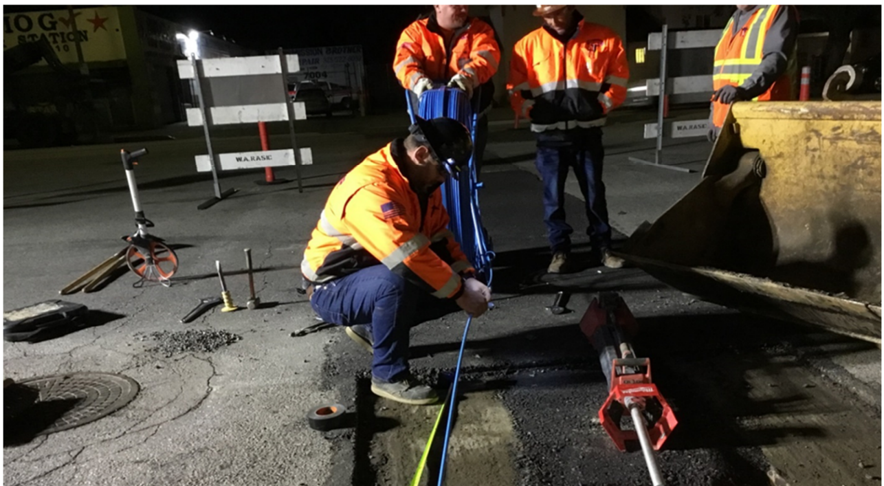
WA Rasic pushed mandrel through conduits 31, 32, 33 and 12. Location: Southbound lanes of Van Nuys Blvd. at intersection of Hart St.
