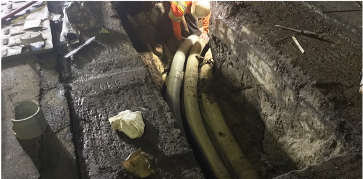
WA Rasic reconfigured orientation of 5" conduits 31, 32 and 33. Location: Northbound lanes of Van Nuys Blvd. at intersecyion of Hart St.
