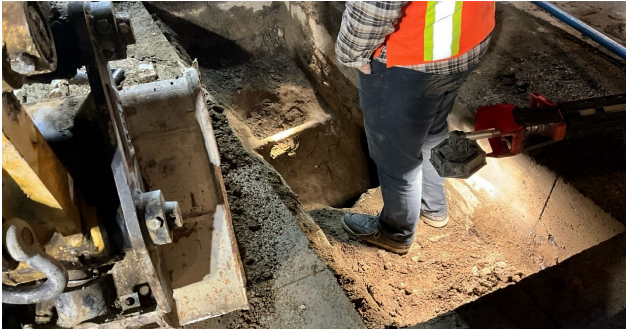
WA Rasic excavated to locate and confirm depth of existing utilities. Location: Northbound lanes of Van Nuys Blvd. at intersection of Vanowen St.
