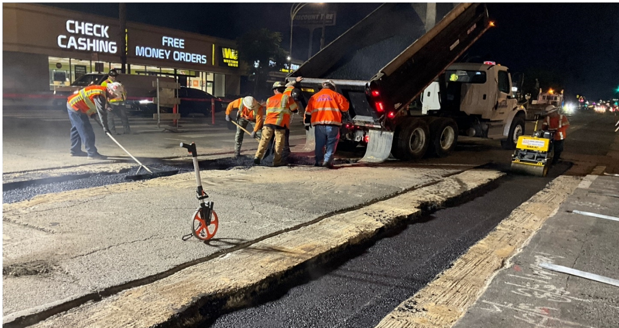
WA Rasic placed asphalt with 4" lifts and compacted. Location: Northbound lanes of Van Nuys Blvd. at intersection of Vanowen St.
