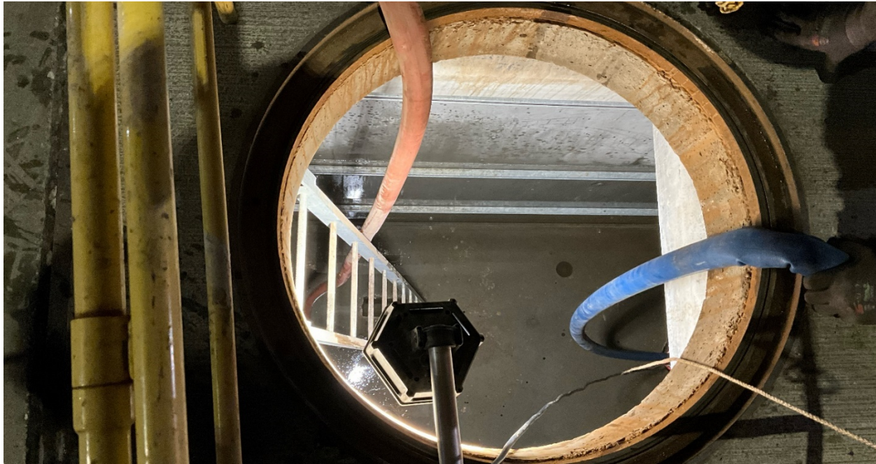
WA Rasic scrubbed inside of vaults and flushed with clean water. Location: Northbound lanes of Van Nuys Blvd. between Hartland St and Hart St.
