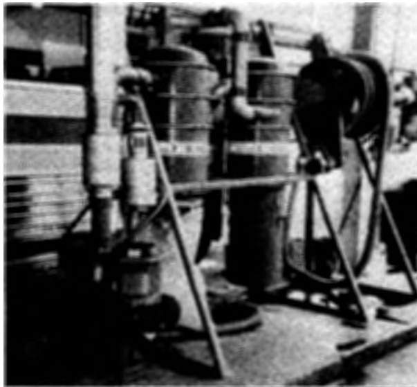
FIGURE 8 Central vacuum system in use at Santa Monica Municipal Bus Lines.
