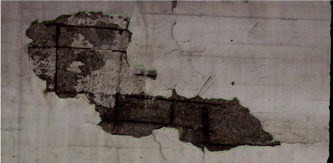
Figure X-7. Closed polyline to determine area of spalling by the ventilation shaft.
