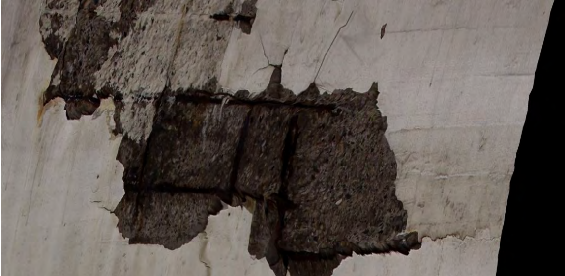
Figure X-4. Foreshortened view of spalling by the ventilation shaft.
