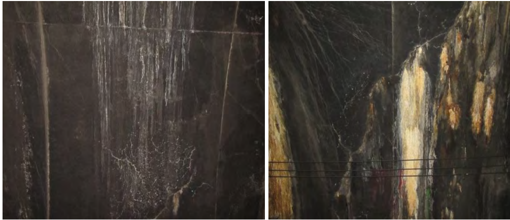
(a) Good condition
