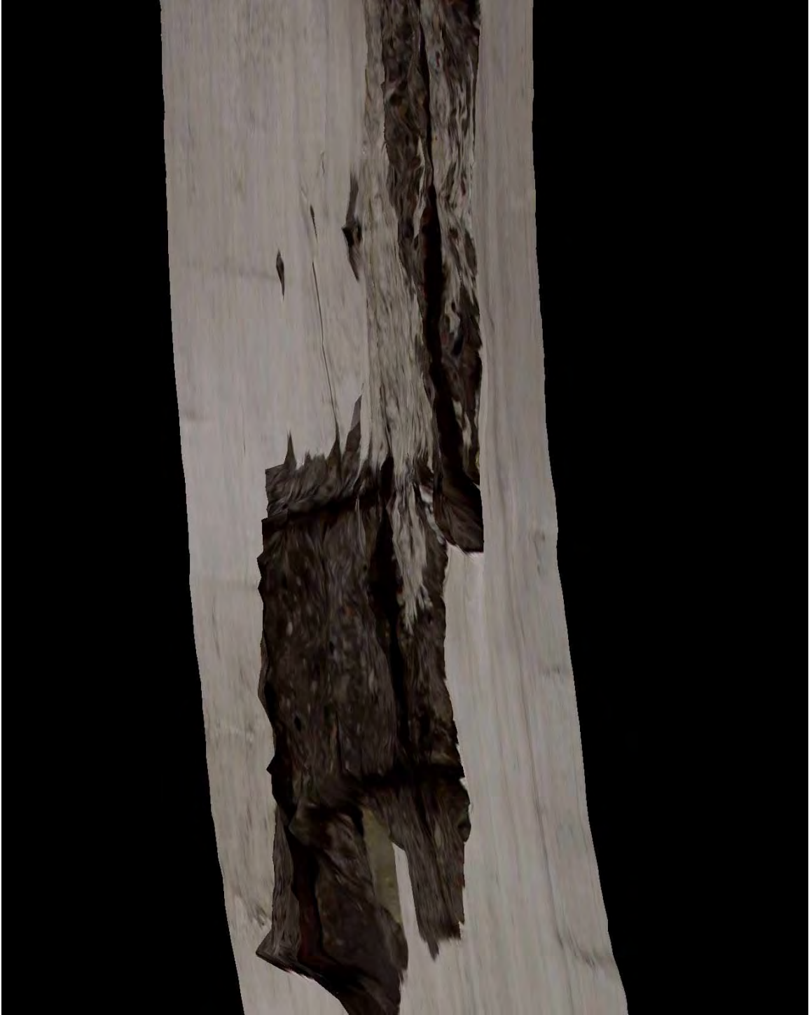
Figure X-6. Backside view of spalling by the ventilation shaft to better appreciate spalling depth and extent.
