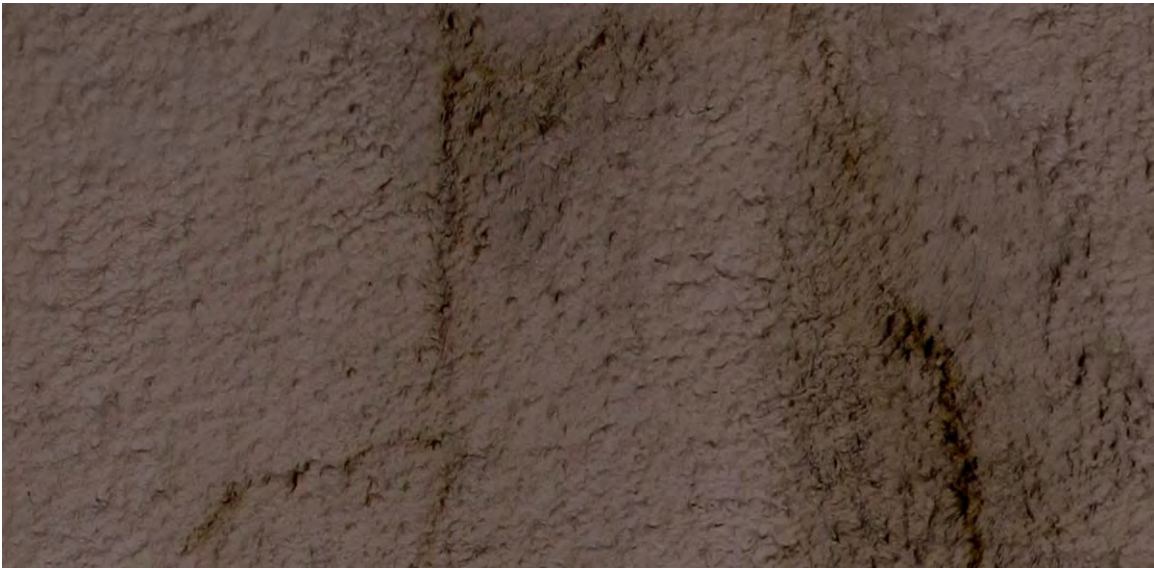
Figure X-12. Detail of shotcrete cracks on left wall by the southern portal with digitized cracks toggled off.
