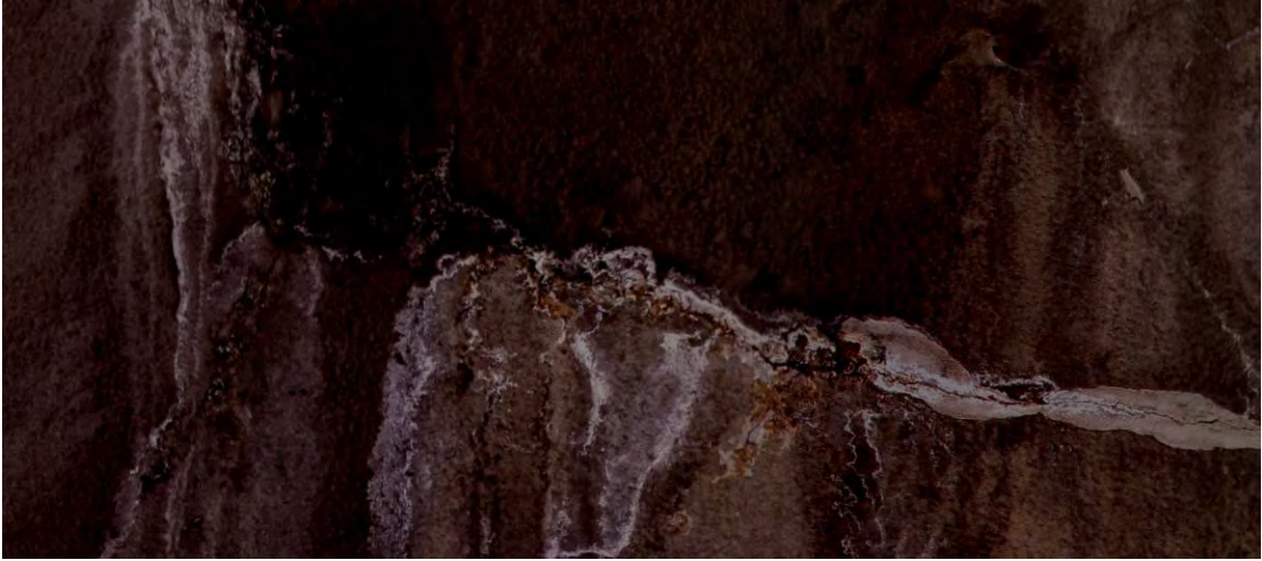
Figure X-21. Eisenhower-Johnson Tunnel: clean air supply duct south-west ventilation building: detail of the south lining wall from within the duct.
