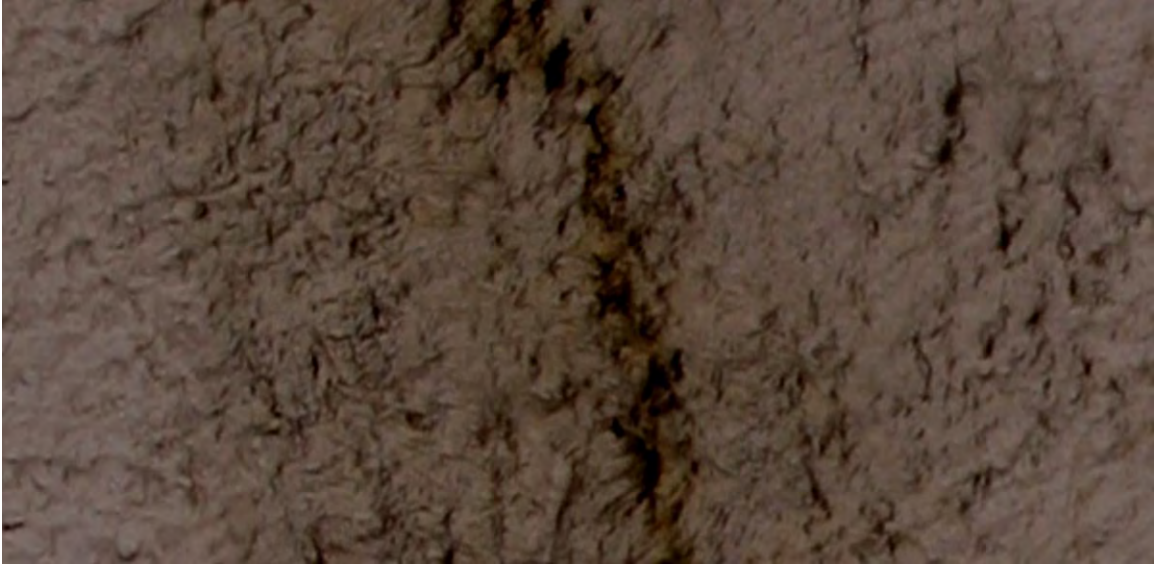
Figure X-13. Close-up view of shotcrete crack on left wall by the southern portal: detail of surface roughness.
