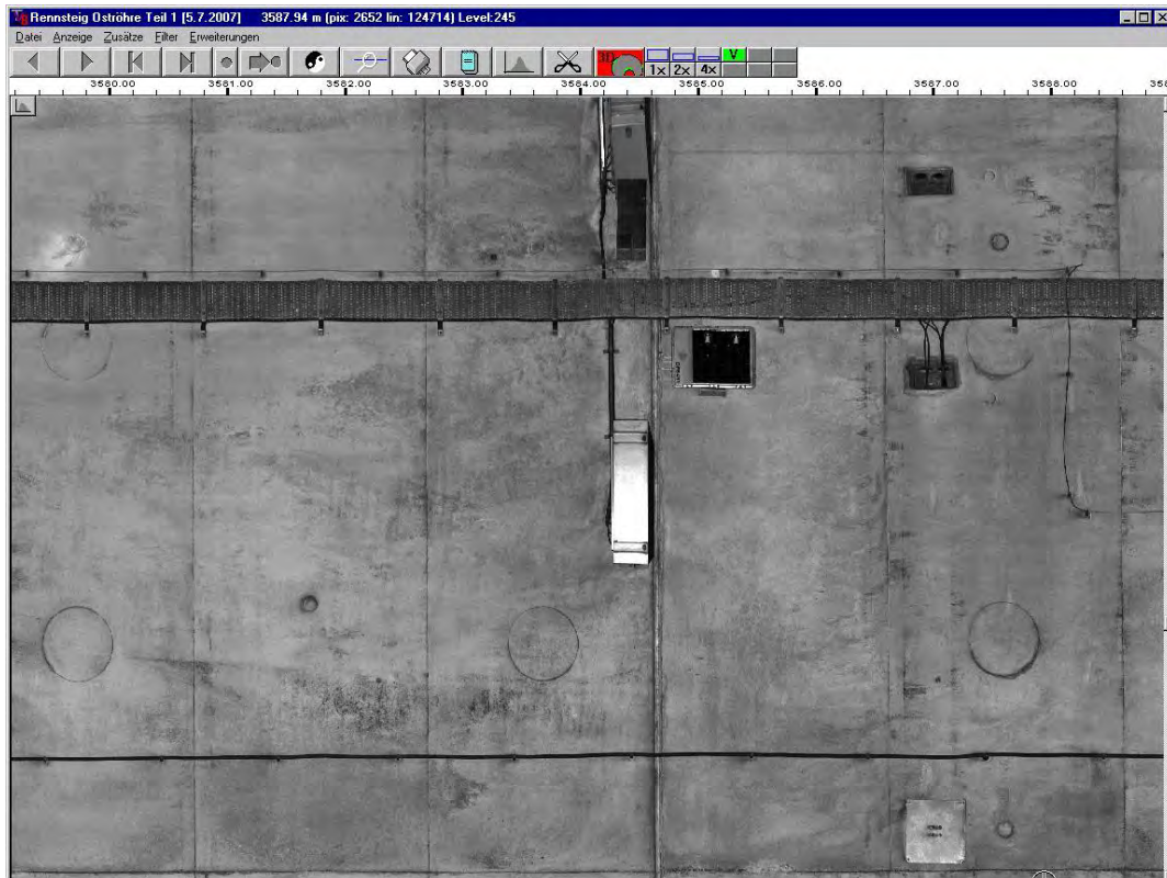
Figure I-3. Visual image showing the conditions of a shotcrete lining in a motorway tunnel.
