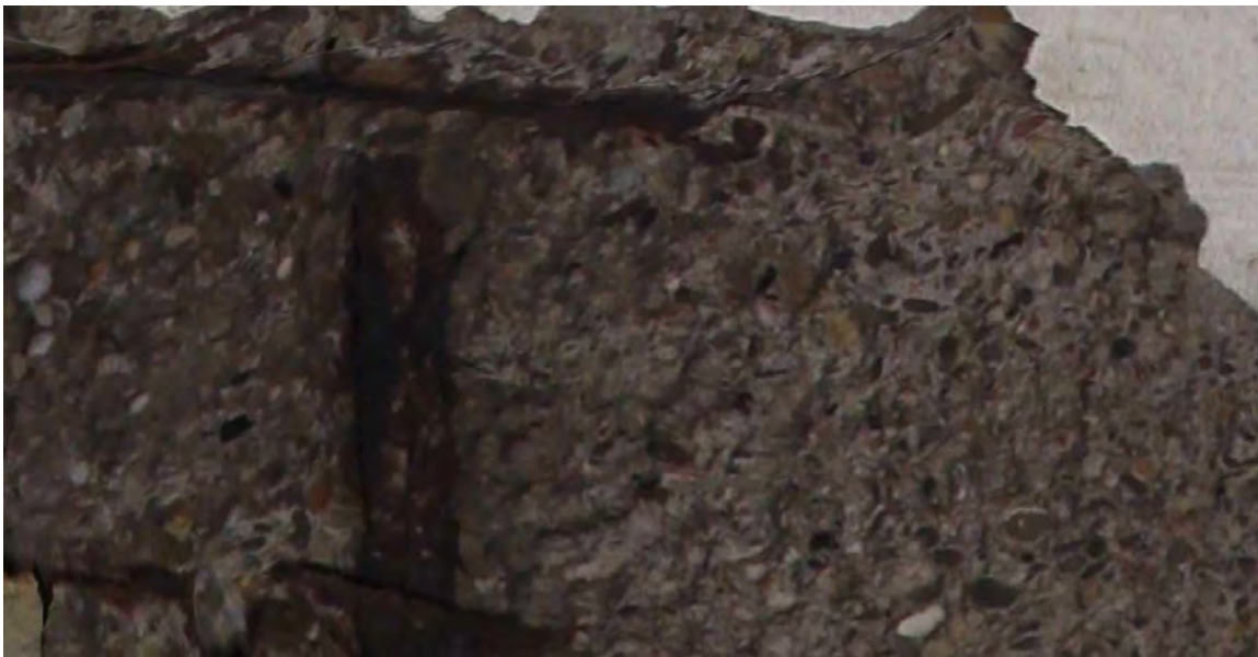
Figure X-5. Detail of exposed aggregate and rebar by the ventilation shaft.
