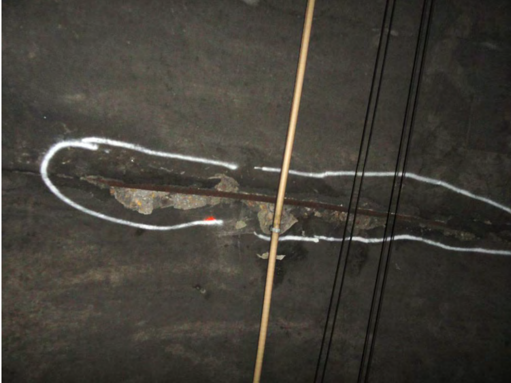
Figure M-47. Typical spalling and corrosion.
