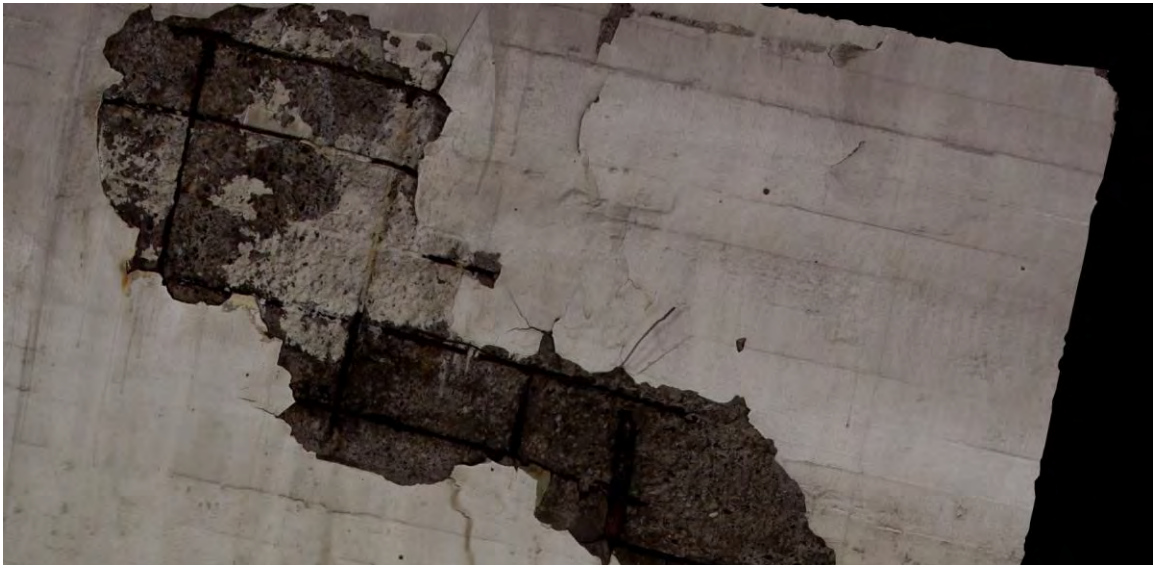
Figure X-3. Detail of spalling by the ventilation shaft.
