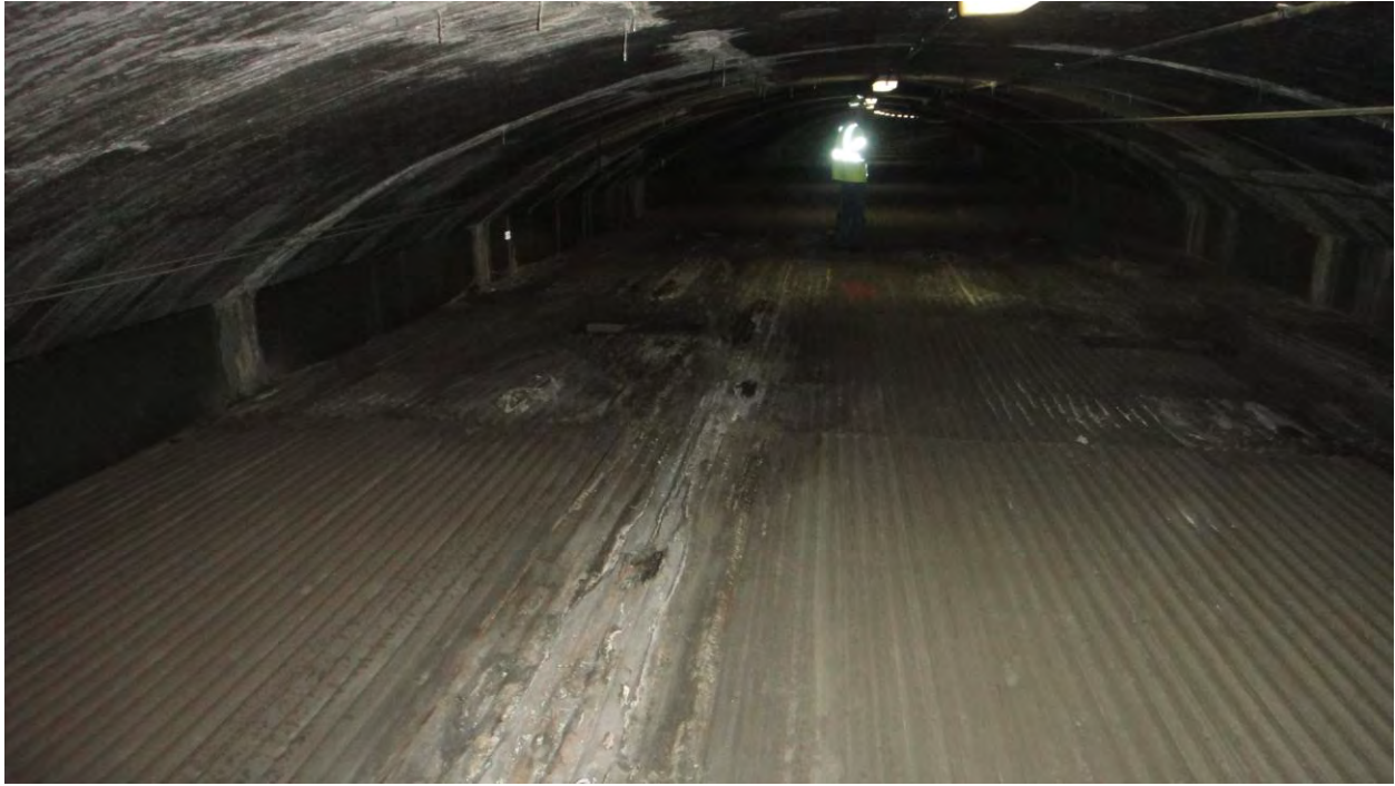
Figure L-25. Visual image of the top of the Hanging Lake Tunnel. Notice the staining around cracks.
