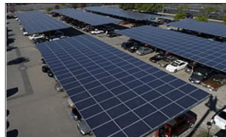
Innovative design includes solar panel array that doubles as a shaded parking area. The energy savings is projected to save the agency $17,000 in energy costs monthly.
