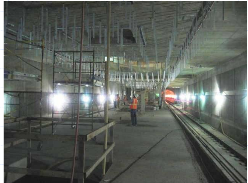
Soto Station – Interior work in the underground rooms progresses as work on the surface structures continues.
