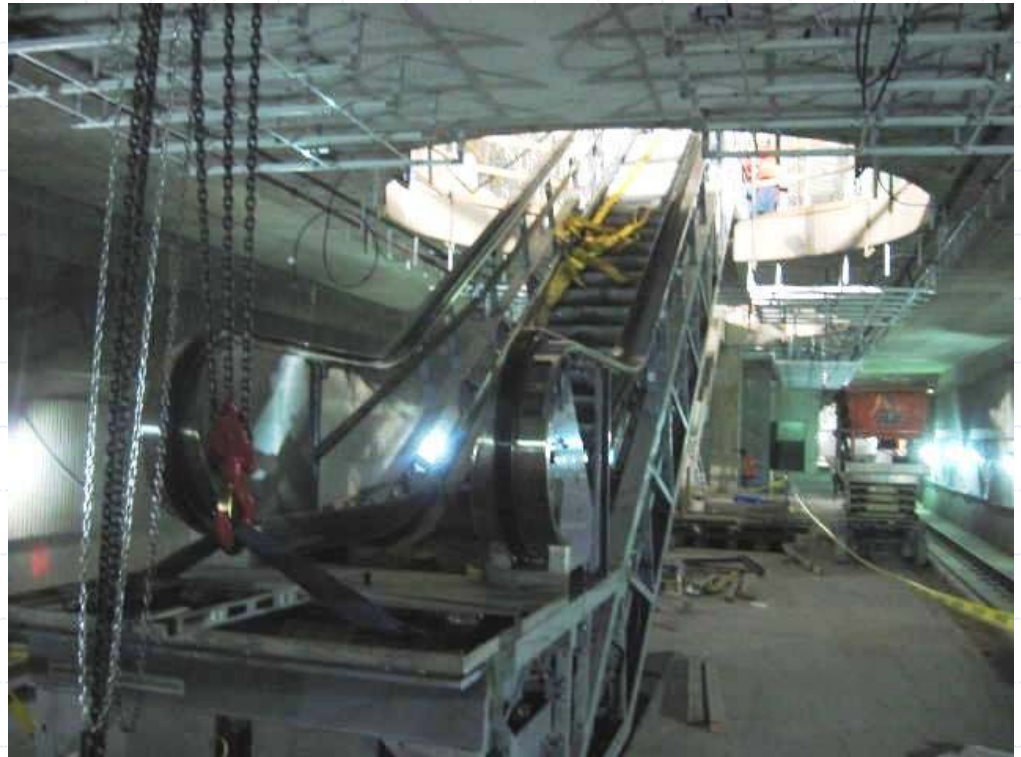
Escalators are being installed to connect the various underground levels. Elevators will be installed within the next few months.
