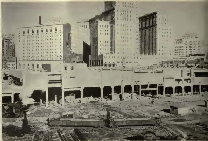
Work is progressing rapidly on the Union Station proper. This view shows a portion of the station construction with its two levels below the street
