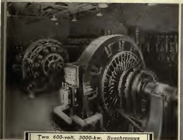
Two 600-volt, 3000-kw. Synchronous Converters and Control Panels, Boston Elevated Railway
