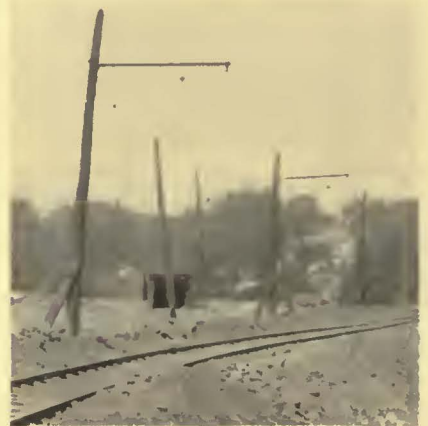
Overhead construction supported by poles mounted on long ties on temporary track at Cleveland
