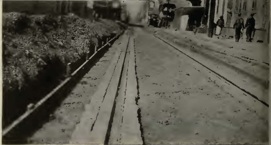
Showing granite blocks placed next to the rails, preparatory to placing the asphalt paving.
