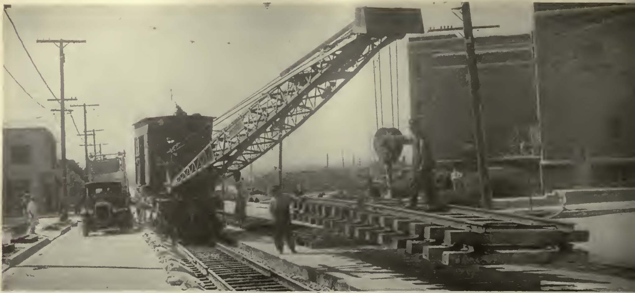
Portable track in 33-ft. sections is placed, removed and carried from one location to another by means of a crane car
