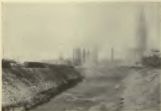
Portion of the Culberson cut, part of the easterly approach to the station. It was necessary to make several large cuts and fills for the electrified right-of-way
