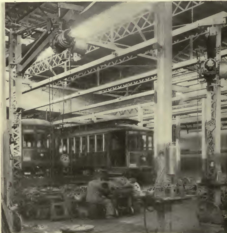
Overhauling motors in the shops of the New Orleans Public Service, Inc. The motor is mounted on a four-wheel carriage which supports it at a height convenient for the workmen
