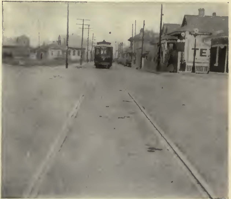
A view of the finished job, protected by Carey Elastite System of Track Insulation. Observe the smooth appearance of the pavement, between the rails and from rails to curb.
