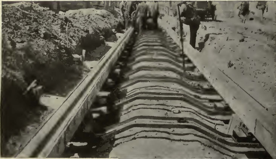
How the New Orleans Public Service, Inc., applied Carey Elastite System of Track Insulation to the inside and outside of the rail. Note the new and interesting type of rail construction in connection with girder rail No. 122-491.
