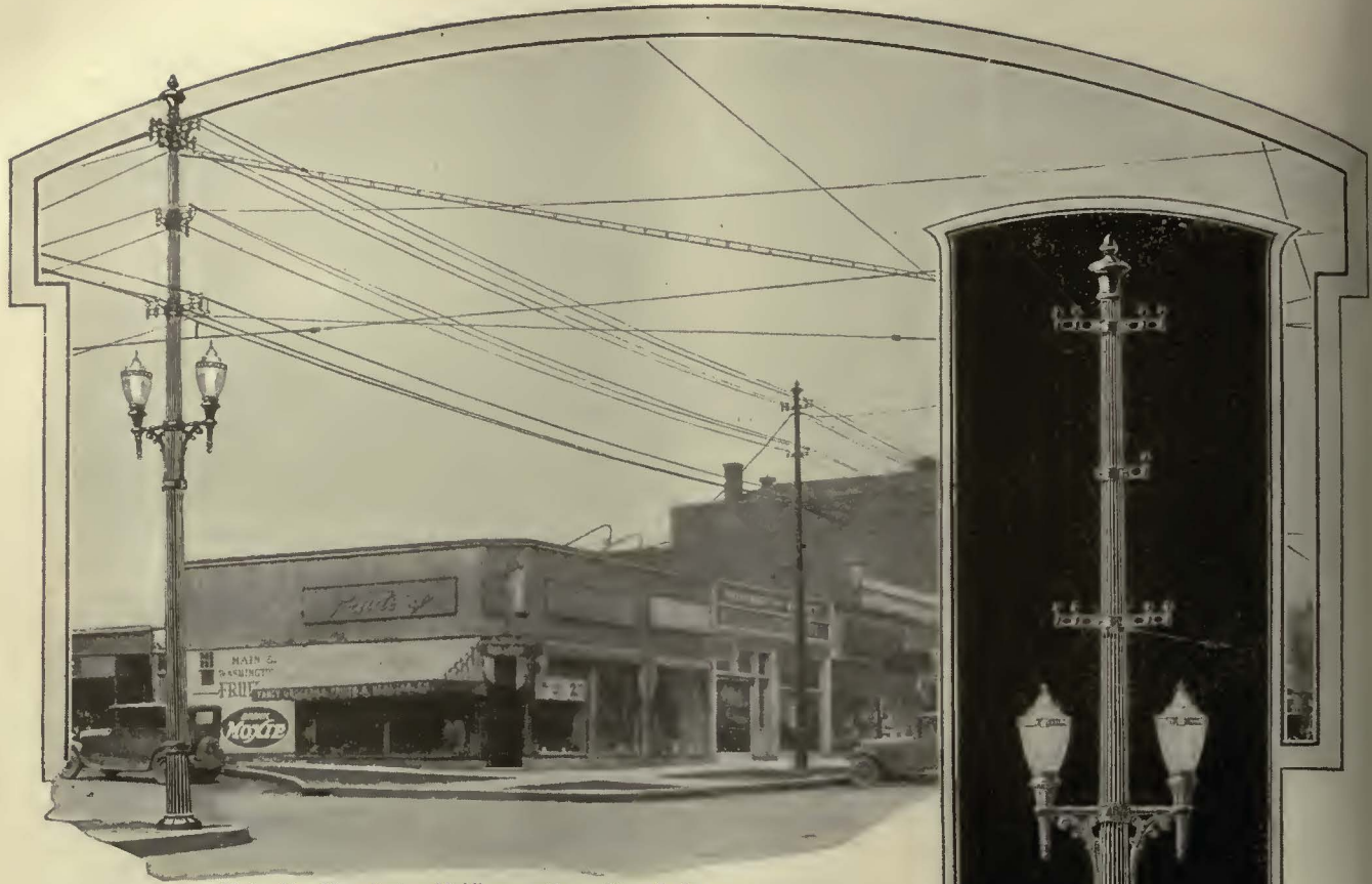
Union Metal installation. Middletown, Conn. Note the heavy loading of the pole at the left.
