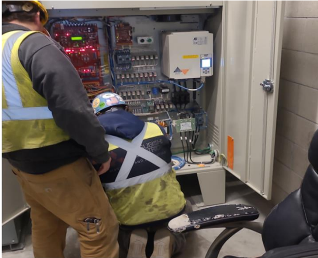
Testing elevator components in the elevator machine room at Little Tokyo/Arts District Station
