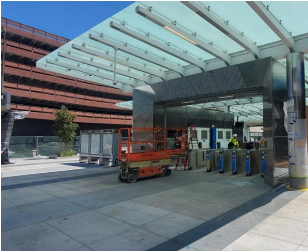
Overview of the western entry portal for the station plaza at Historic Broadway Station
