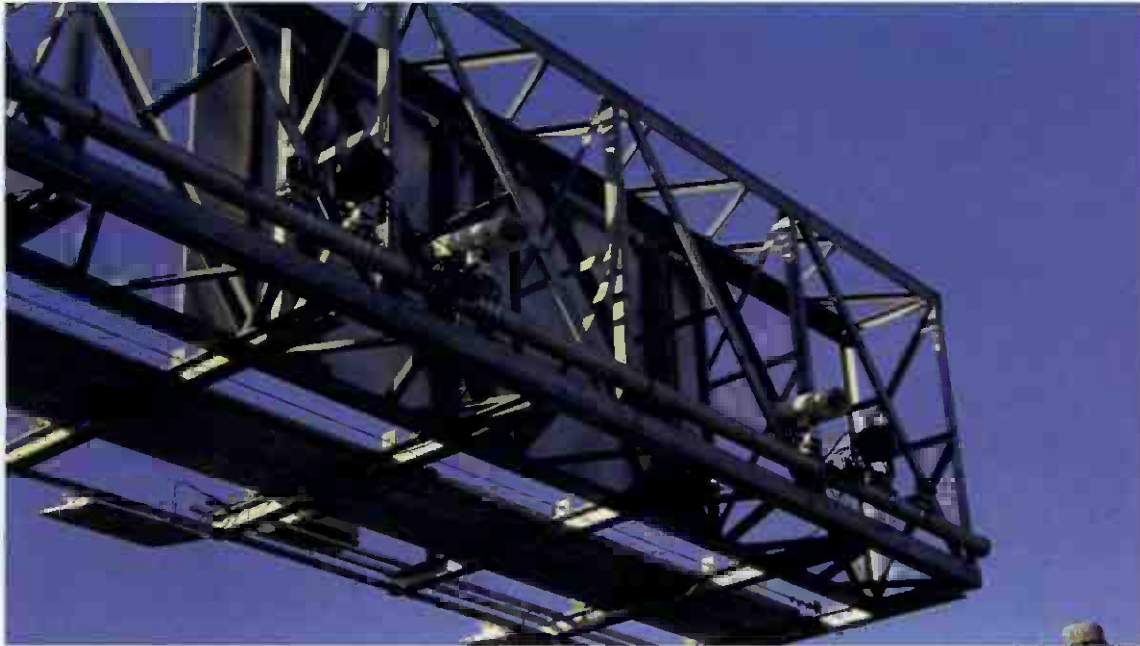
DSC 1133 new camera's installed on overhead sign on I-110.
