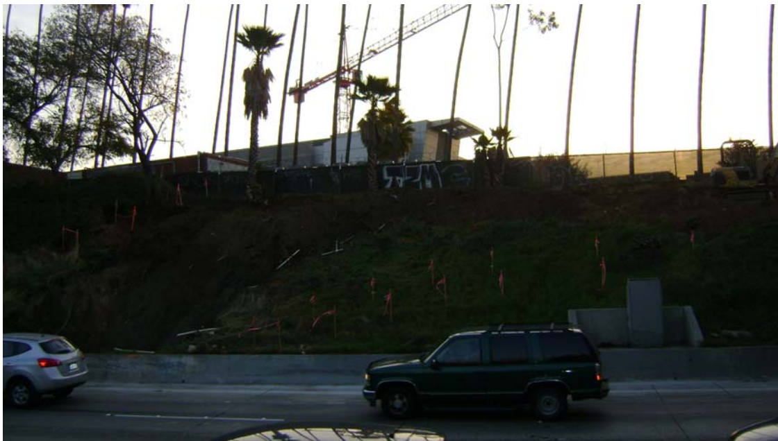
Removing ADL [material containing aerielly deposited lead] at the foundation area of the new POC.
