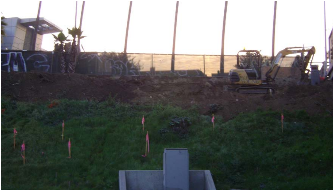
Heavy equipment starting the excavation for the new pedestrian over crossing located at Adams Blvd.
