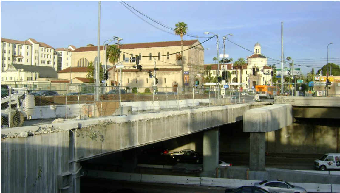
Demo-work on the Adams Bridge over the I-110 in order to start the Bridge Widening.
