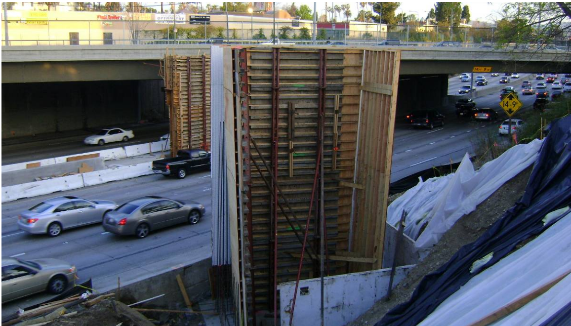
Form work in place for the East Wall support for the new Pedestrian Overcrossing on the I-110.
