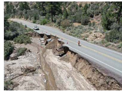
State Route 38 Storm Damage
