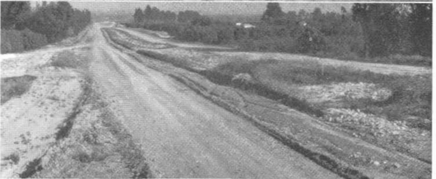
UPPER—Looking northerly along construction toward end of job at First Street Overcrossing. CENTER—Looking southerly along construction from top of fill for Newport Avenue Undercrossing. LOWER—Looking southerly on construction from fill for Route 2/43 separation at Tustin Avenue.
