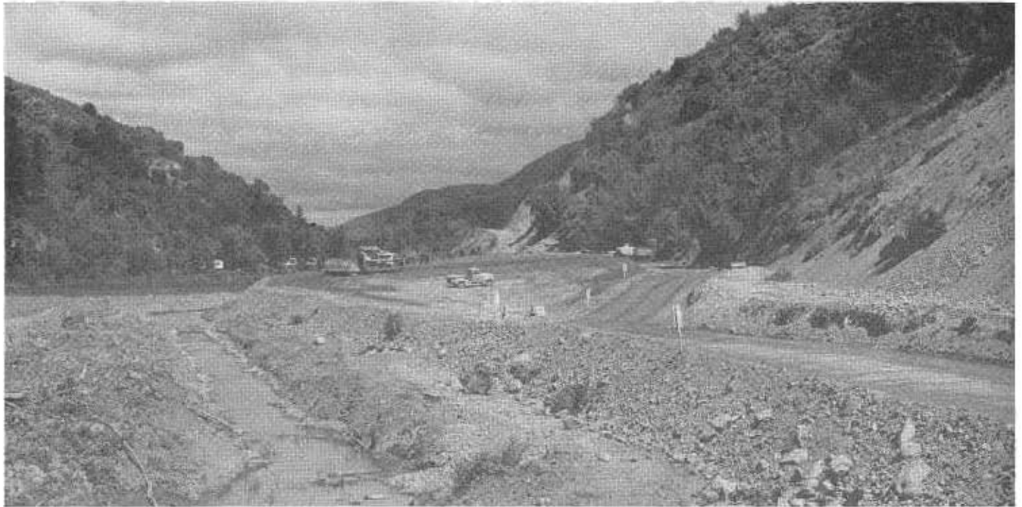
Looking westerly at construction activities on Laurel Dell-Tule Lake project in Lake County at intersection with Scotts Valley Road and at easterly end of Laurel Dell Lake.
