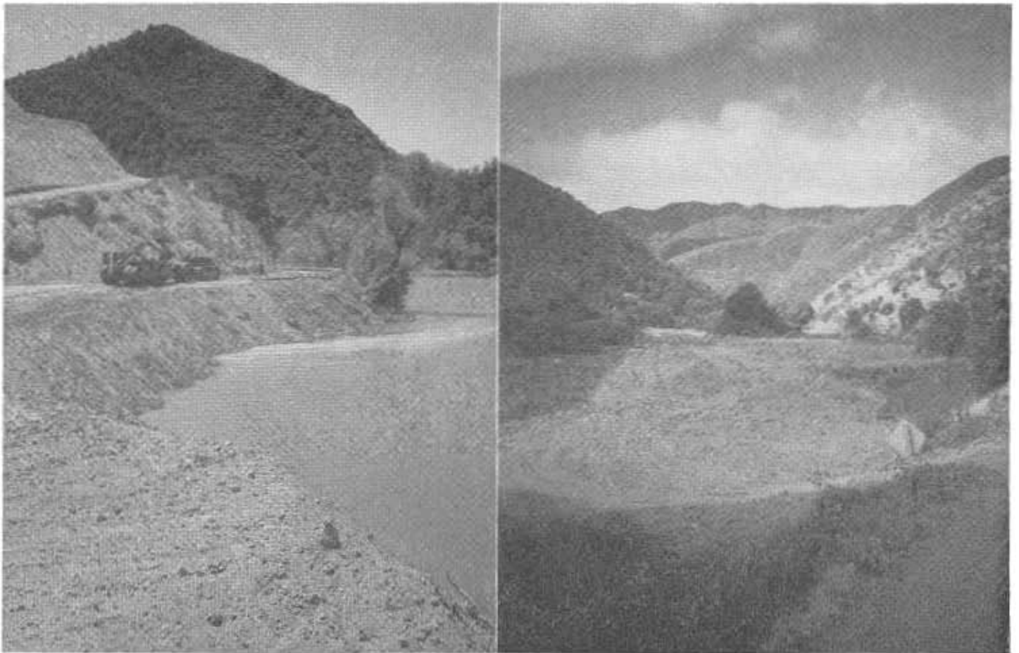
LEFT—Looking easterly along shores of Laurel Dell-Tule Lake project. Note sharp, narrow turn on old highway that will be superseded by new, modern alignment. RIGHT—Looking westerly along new grade on the Laurel Dell-Tule Lake project. New alignment replaces narrow, winding old highway which turns off to right and follows along base of hills forming the Scotts Creek Canyon.
