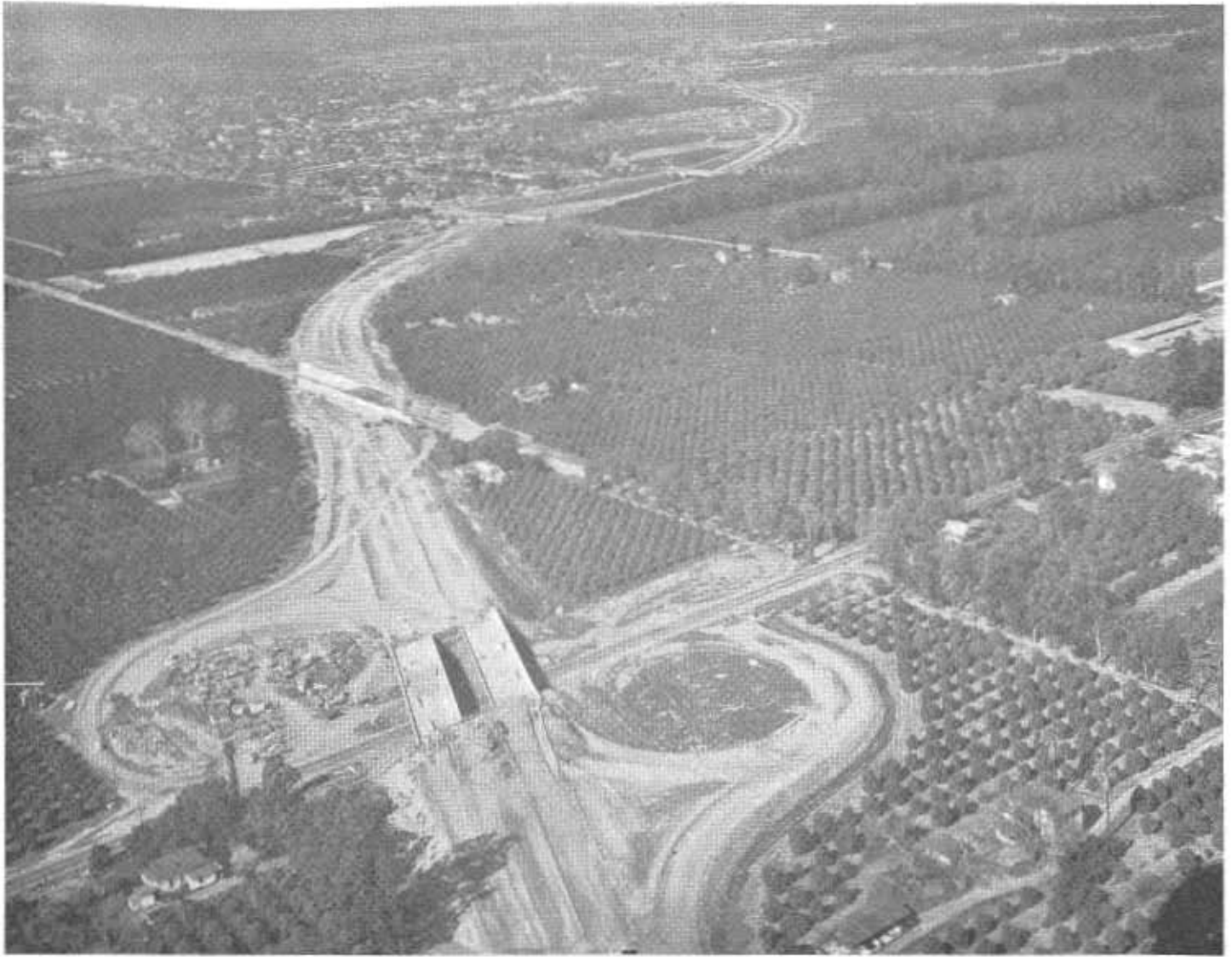
Looking northerly on Santa Ana Freeway from Tustin Avenue to First Street. The completed Route 2/43 separation structure is shown in foreground.
