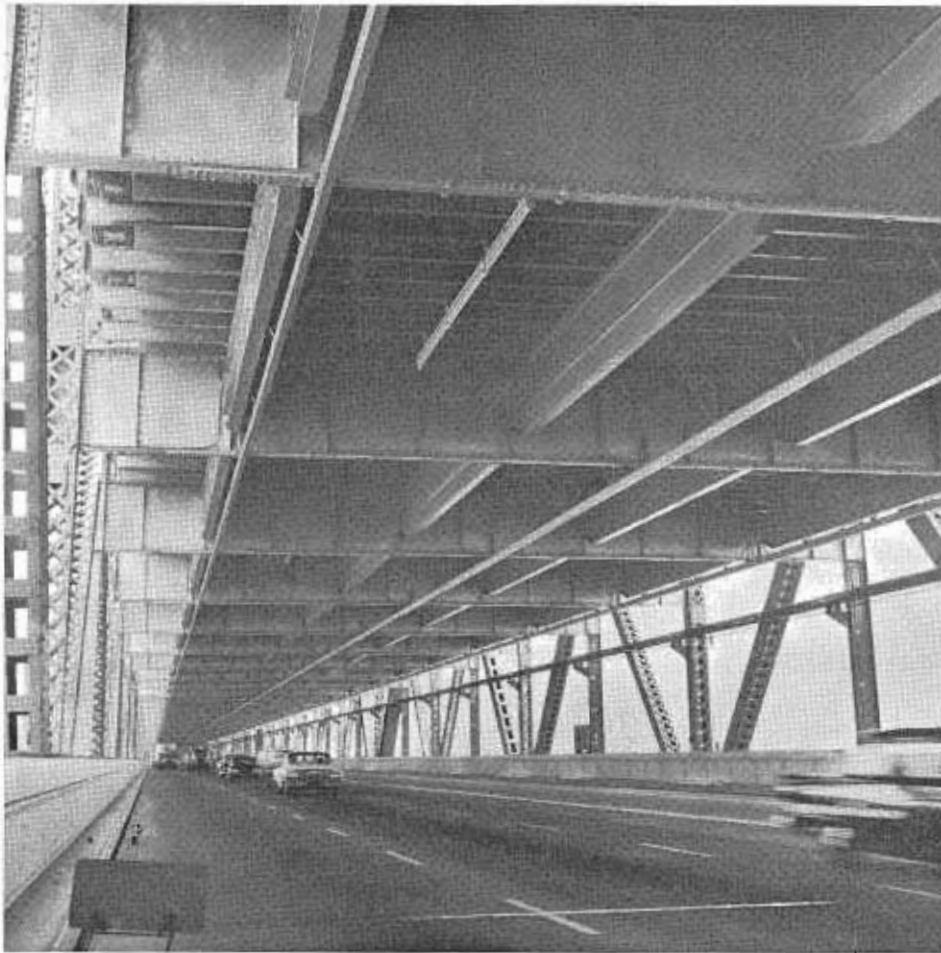
The completed upper deck strengthening as seen from below on the lower deck showing the additional transverse joists, understringers, floor beam coverplate and typical lower deck lighting installation.
