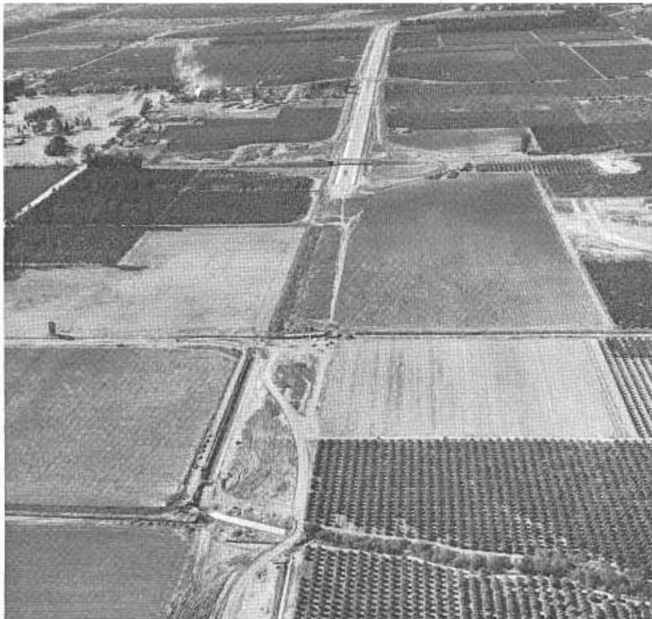
The Route 126 Freeway is under construction northeastward from Saticoy to Santa Paula through the Santa Clara River valley in Ventura County. This 8.5-mile project, under contract for nearly $7,000,000, will be completed in mid-1965. This view is westward along the completed section toward Ventura.
