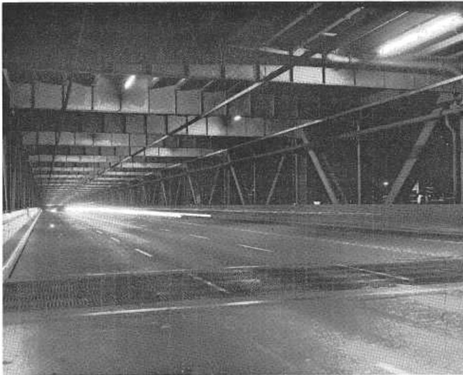
Lower deck lighting on the West Bay spans.
