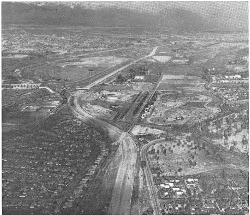
Looking south along the San Gabriel River Freeway under construction. Rose Hills Road crossing is in center, and Whittier Narrows Dam is at the left.
