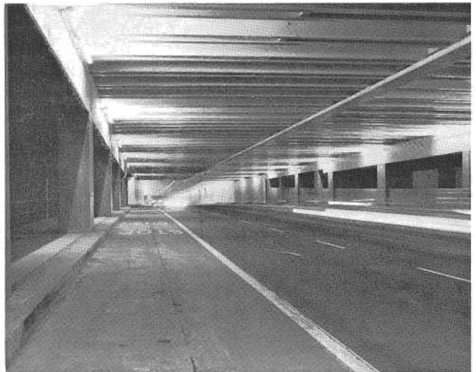
Lower deck lighting on the viaduct section of the East Bay spans looking west toward the tunnel.
