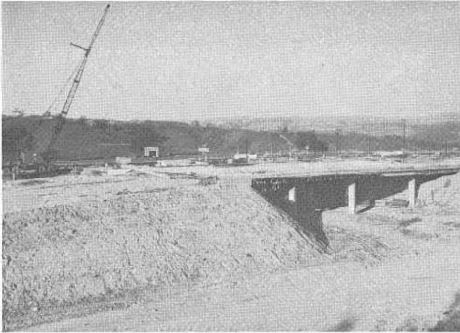
An interchange between the Golden State Freeway and the future Route 126 Freeway is under construction at Castaic, on the Ridge Route north of San Fernando. The project is part of a program to improve the Golden State (Interstate Route 5) to full freeway standards between San Fernando and the Kern county line.
