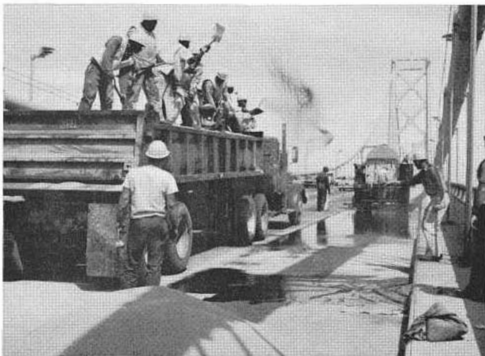
Equipment train for resurfacing the upper deck. The special truck for placing 1/8-inch-thick epoxy coal tar is in the lead followed by fine aggregate truck.
