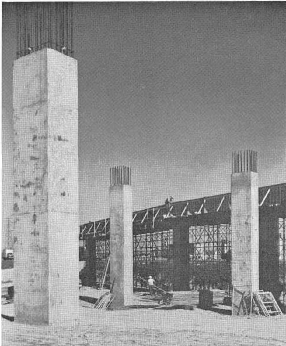
These massive columns will support a structure of the interchange between the Santa Ana and San Gabriel River Freeways, now under construction in the Santa Fe Springs area.
