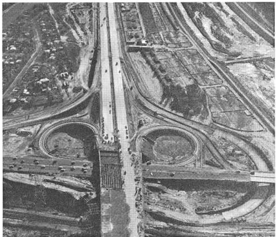
Interchange begins to take shape at Valley Boulevard as the San Gabriel River Freeway construction is being pushed in southeastern Los Angeles County.
