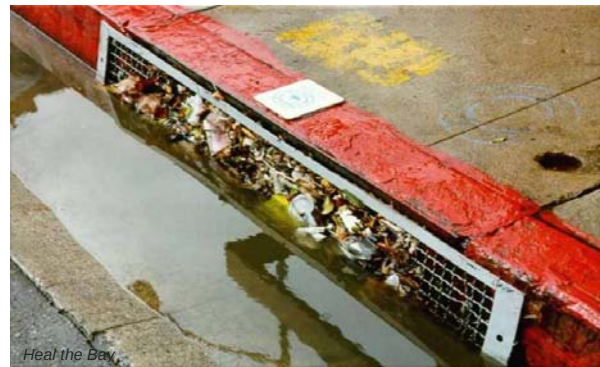
A clogged catch basin in Los Angeles.
