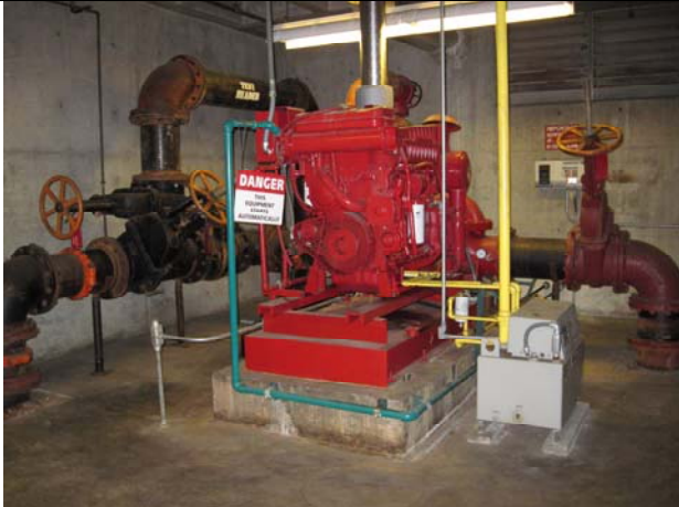
PHOTO O: View of a typical on-site Fire Pump
