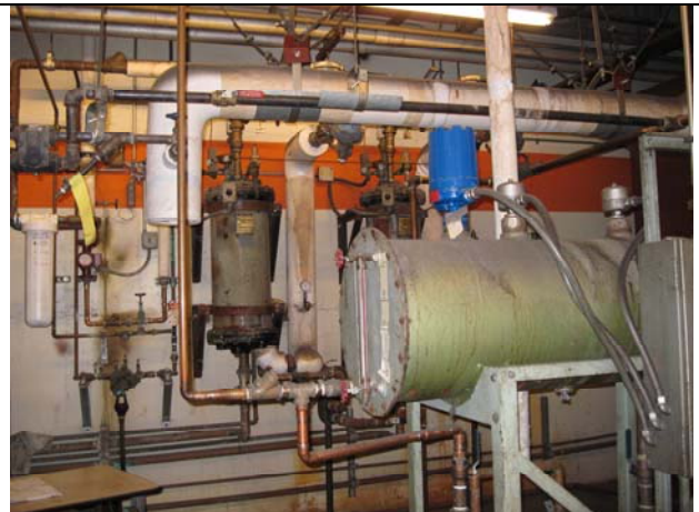
PHOTO R: View of a boiler on the ground floor of the West Hall
