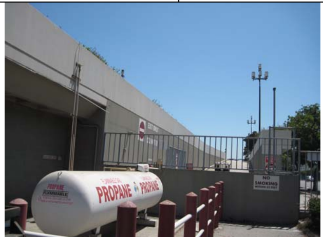
PHOTO L: View of the on-site propane AST, located at the exterior of the northwestern portion of the West Hall
