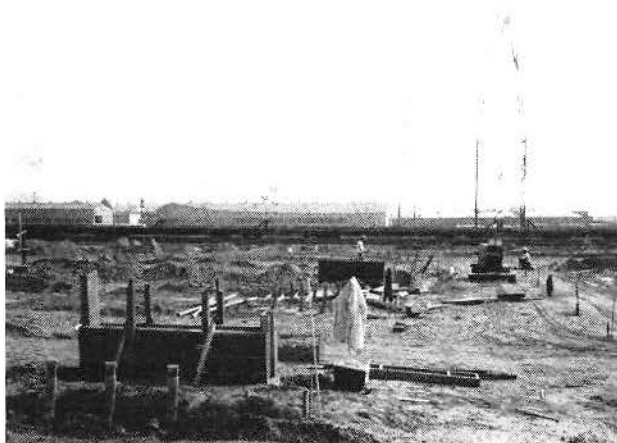
TRACTION POWER STUBUPS, EAST OF MOW BLDG.
