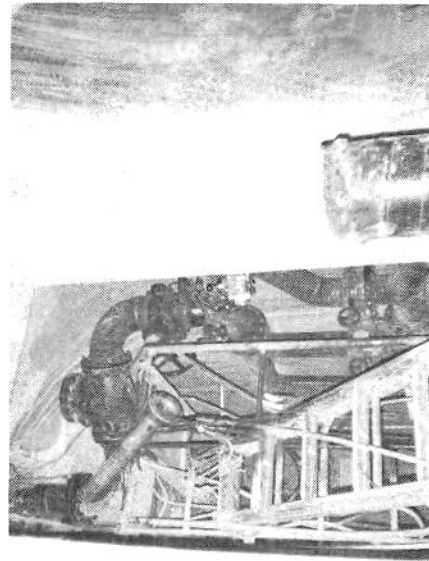
WET STAND PIPE SUPPLY LINE IN CROSSPASSAGE 12
