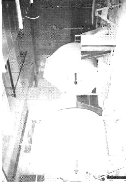
DISTRICT FURNISHED FANS IN FAN ROOM #61 IN THE HOME SAVINGS BLDG.
