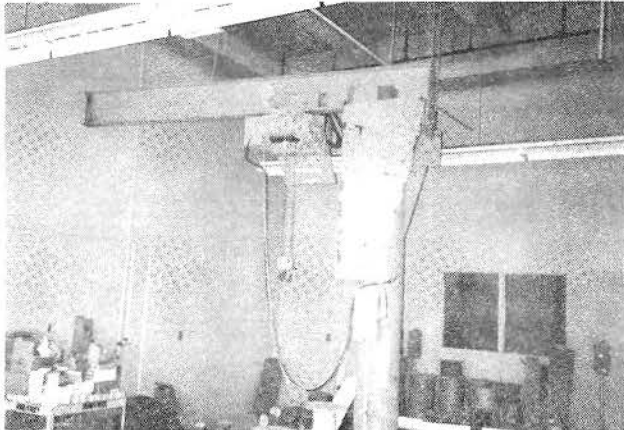
JIB CRANE INSTALLED IN THE METALS SHOP
