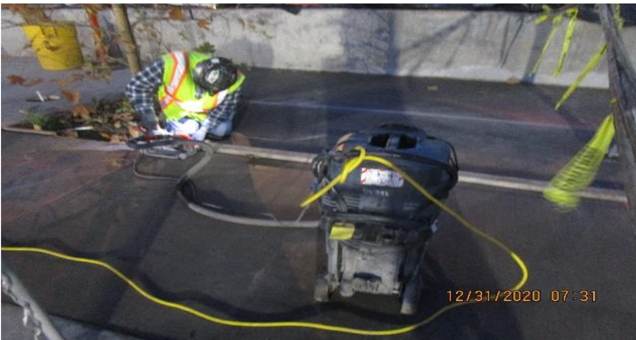
EXPO STATION– Saw cutting control joints for the architectural topping slab at the north side of the plaza.
