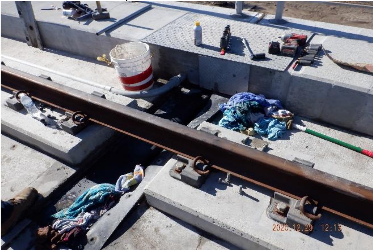
AVIATION/CENTURY- STA 72+10 TK#3/SB looking west – Century Bridge deck joint dismantle , cleaning rubber seal to address leaking
