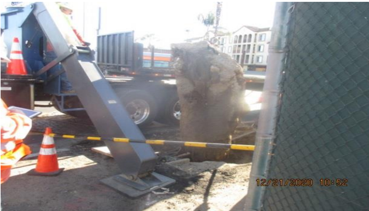
PARK MESA – Continue removing existing street light foundation on the southwest corner of 60th St and Crenshaw Blvd.
