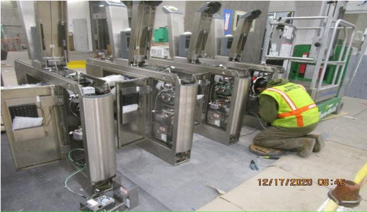
UG3 – Vernon, between Free Area C129 & Paid area C146 terminating #12 load conductors & CAT-6 data.
