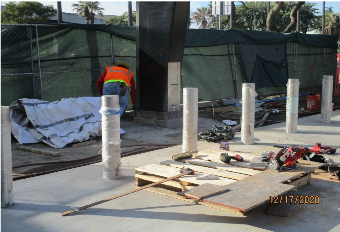
AVIATION/CENTURY- Setting forms for the hardscape concrete at the SW corner of Aviation and Century.
