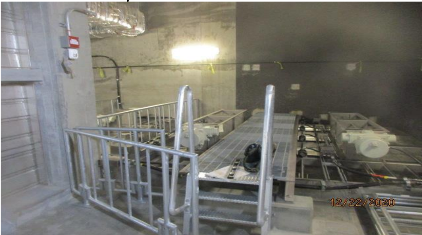
LEIMERT PARK STATION – Drilling and setting guardrails around the dampers inside the Emergency Ventilation Shaft/OTE Plenum North C-127 and South C-101.
