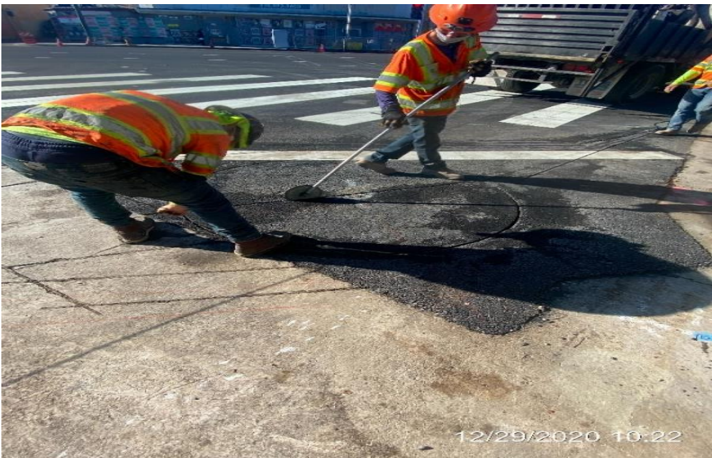
LEIMERT PARK STATION – Saw cutting pavement for vehicle detection loops on northbound Crenshaw Blvd and 43rd Pl.
