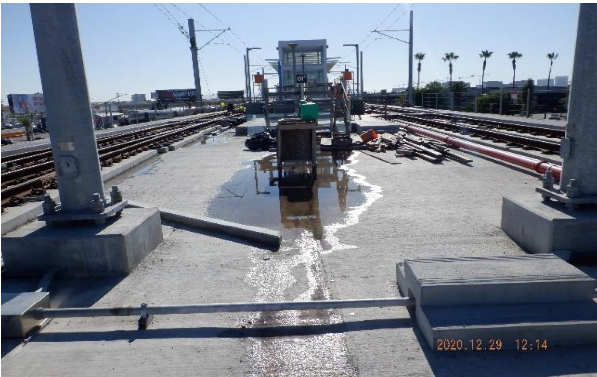
AVIATION/CENTURY- STA 71+00 looking south – water pond on Century Bridge deck's.
