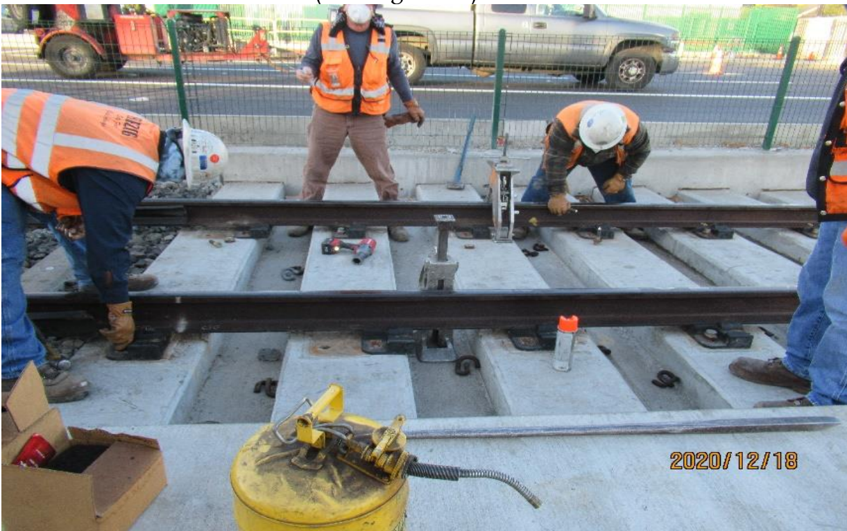
PARK MESA – HCC on NB track at 48th Street, removing DF fastener plates for investigation of potential loose inserts STA 364+48 (looking West)
