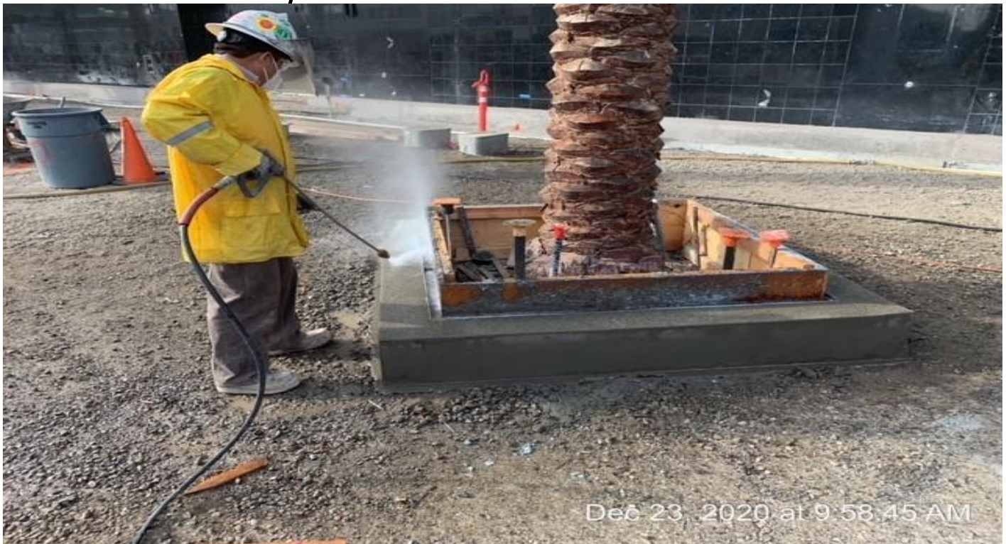
MLK STATION – Removing formwork and power washing top cast paste from palm tree and pedestrian light poles bases at the plaza.
