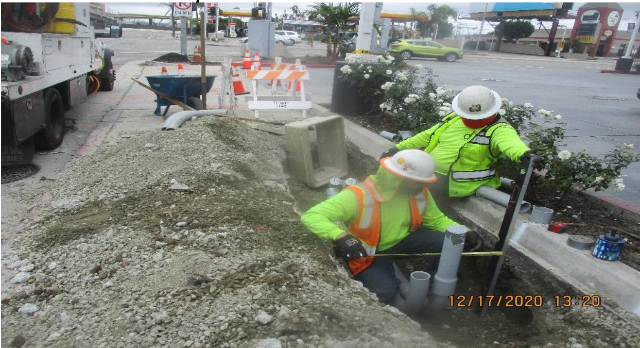
AVIATION/CENTURY- DB Electric Place conduit to controller location at Century and Aviation.
