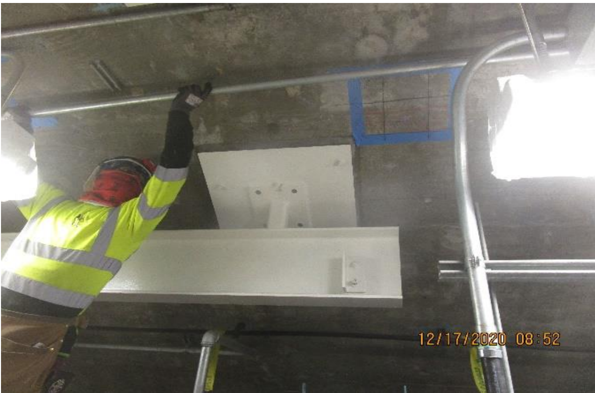
UG3 – Vernon Concourse, Ejector room C134, begin re-pipping 1" GRC from ejector control panel Vernon-SE-6-2XC
