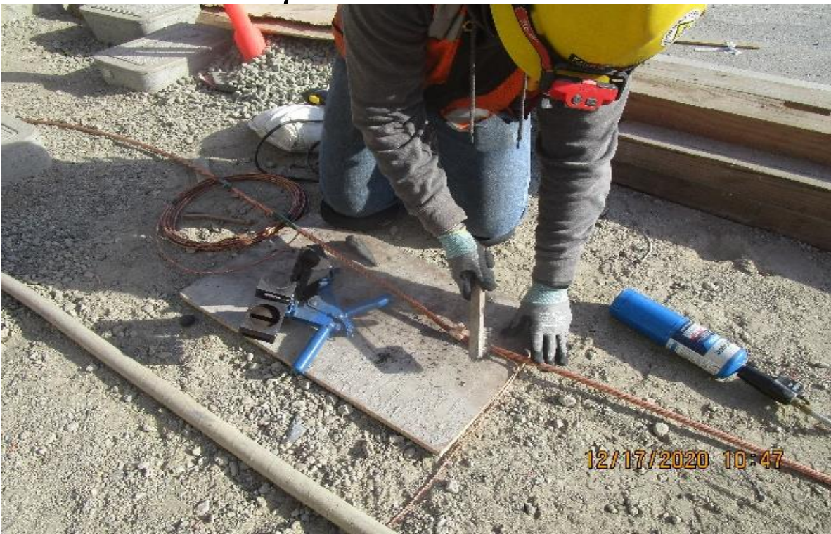
MLK STATION – MLK (S) Plaza, Continued CAD welding #6 aux grounds from 4/0 bare copper CU grounding grid for bicycle racks
