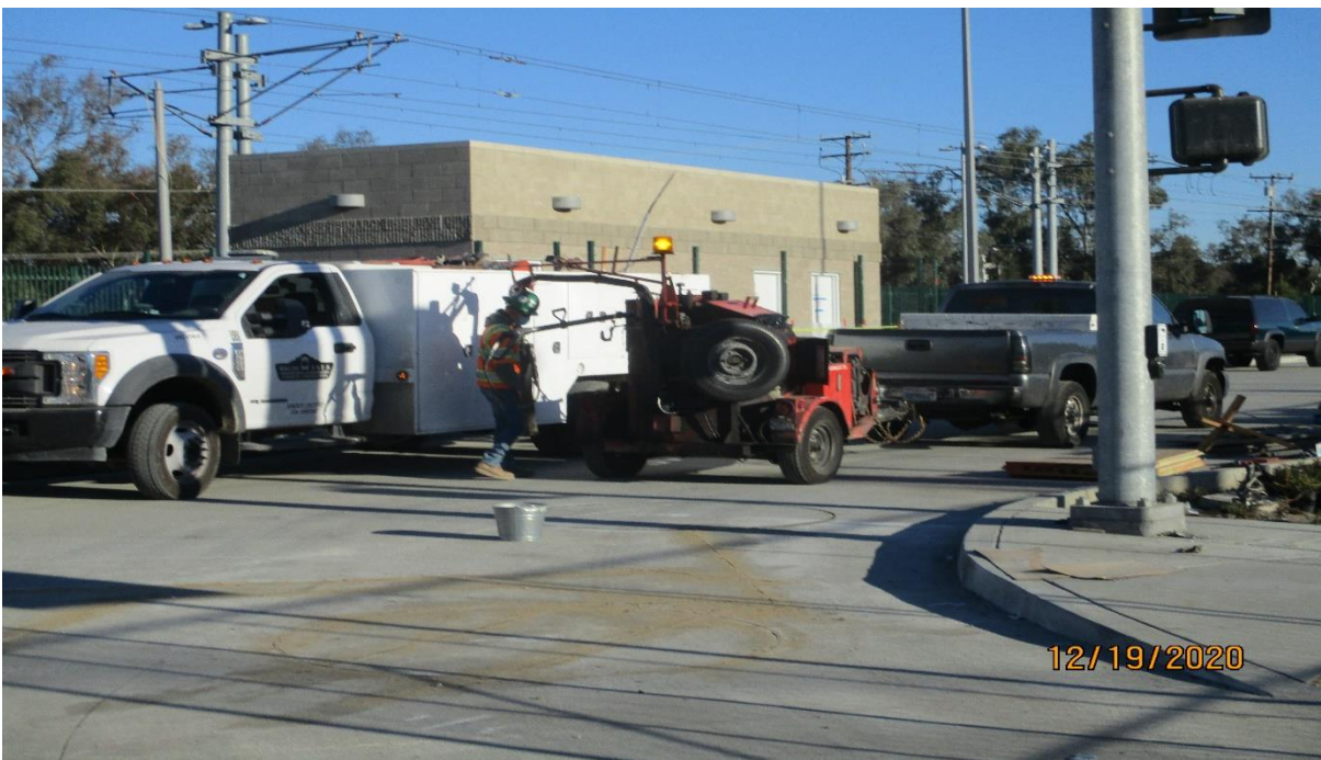
La Brea Station - Traffic loop detector installation at the La Brea Station.
