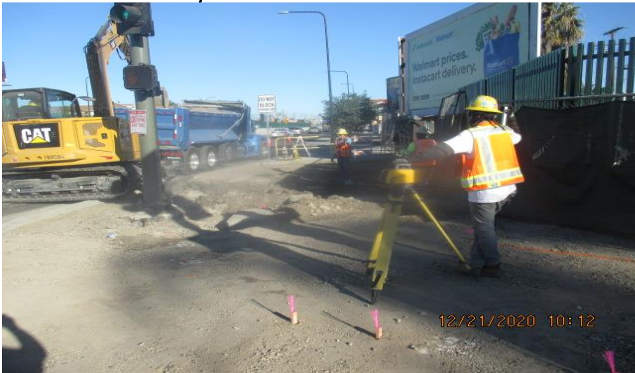
PARK MESA – Excavating/grading for new sidewalk and ADA ramp installation on the northwest corner of 60th St and Crenshaw Blvd.
