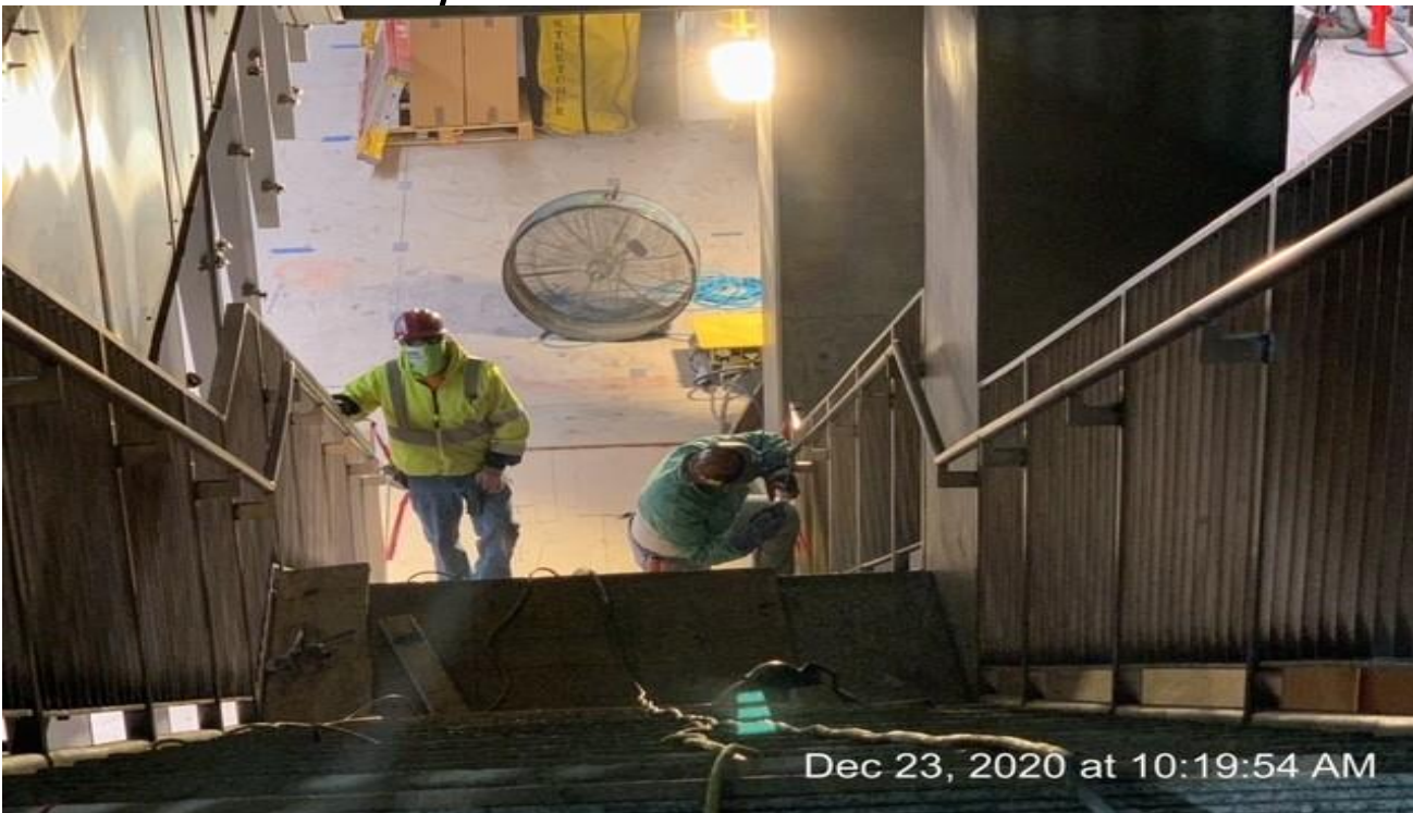
MLK STATION – Fastening and welding handrails to the guardrails of Staircase 3 from concourse to platform.
