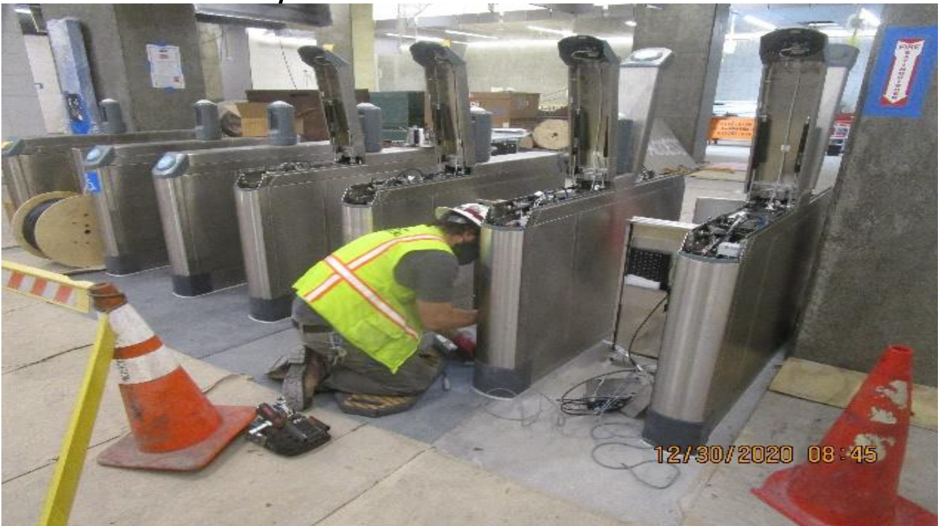
LEIMERT PARK STATION – Continue performing electrical work to the Fare Gate/TVM system at the Paid & Free Area.
