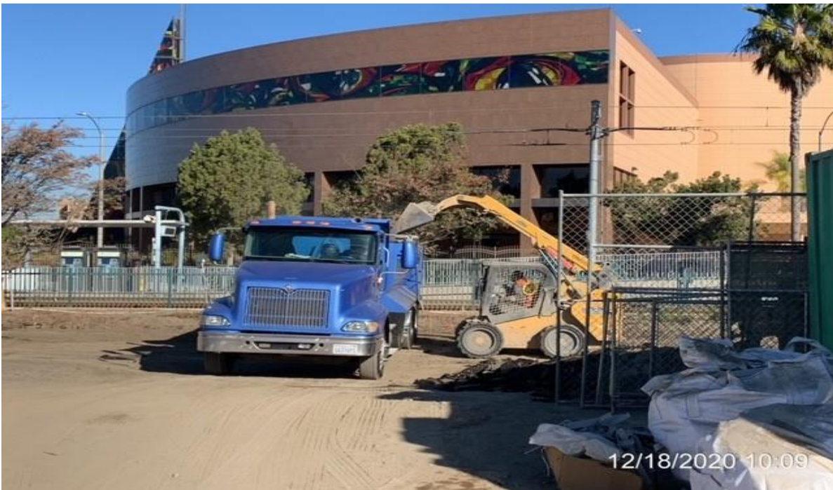
EXPO STATION - Removing and loading out demolished asphalt concrete at the north side of the plaza.
