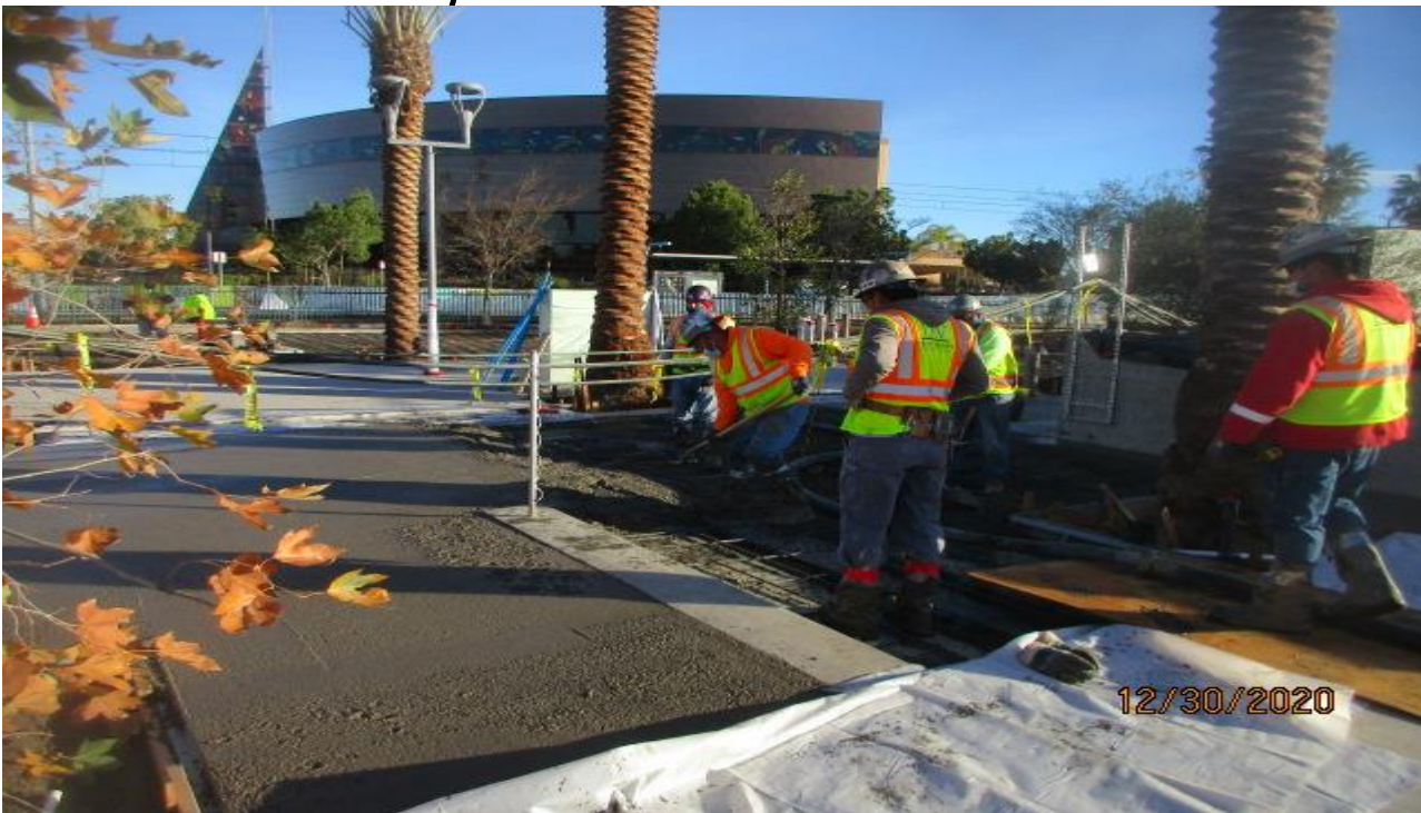
EXPO STATION– Continue placing concrete for the architectural topping slab at the north side of the plaza.
