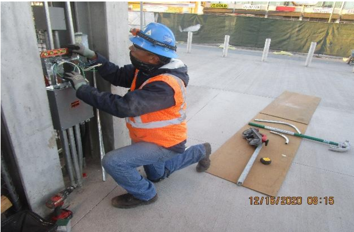
UG3 – Vernon Plaza, GLs 13.8,D, pulling #12 XHHW-2, hot, neutral, grounds switches (3) Metro illuminated disc signs.
