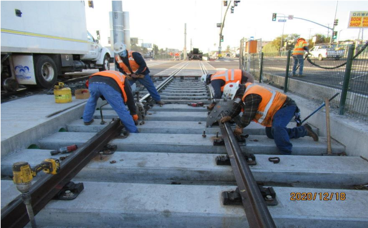
PARK MESA – HCC at 48th Street SB track verifying potential loose inserts on Baffle plinths STA 364+48 (looking south)
