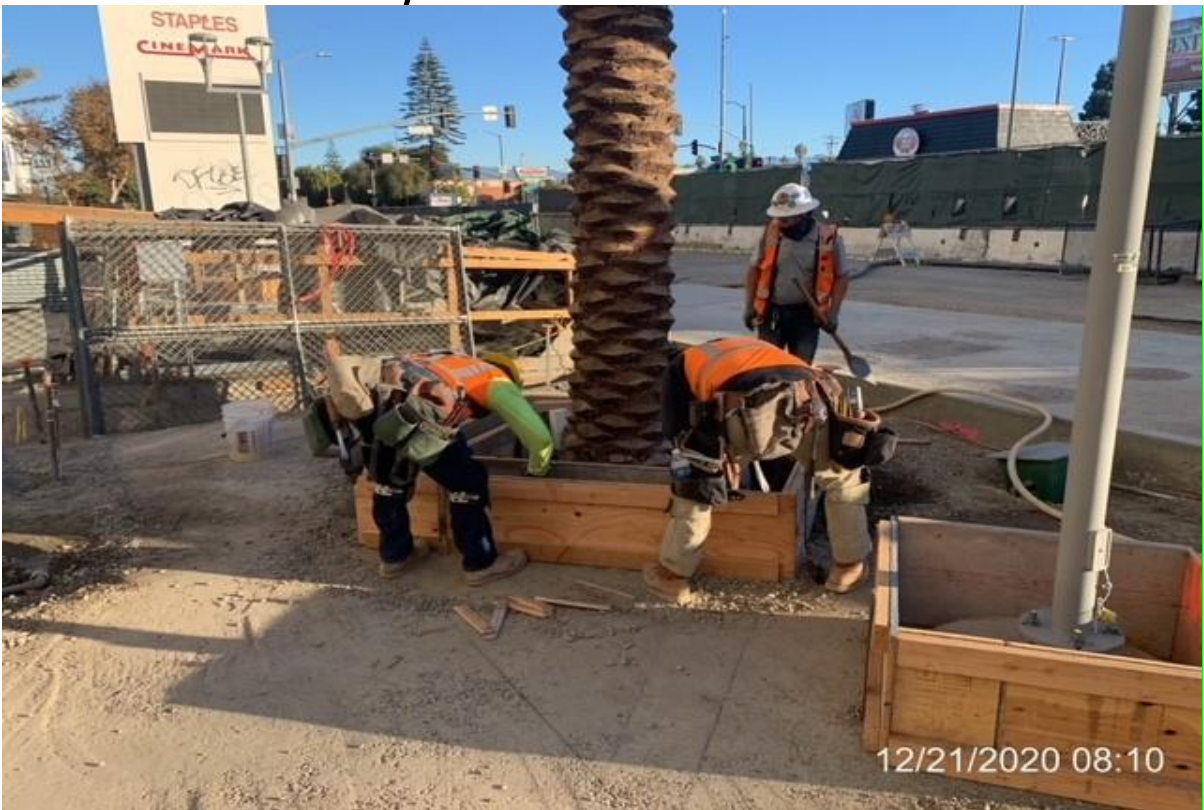
MLK STATION – WSCC carpenters at plaza level setting formwork for tree bases.
