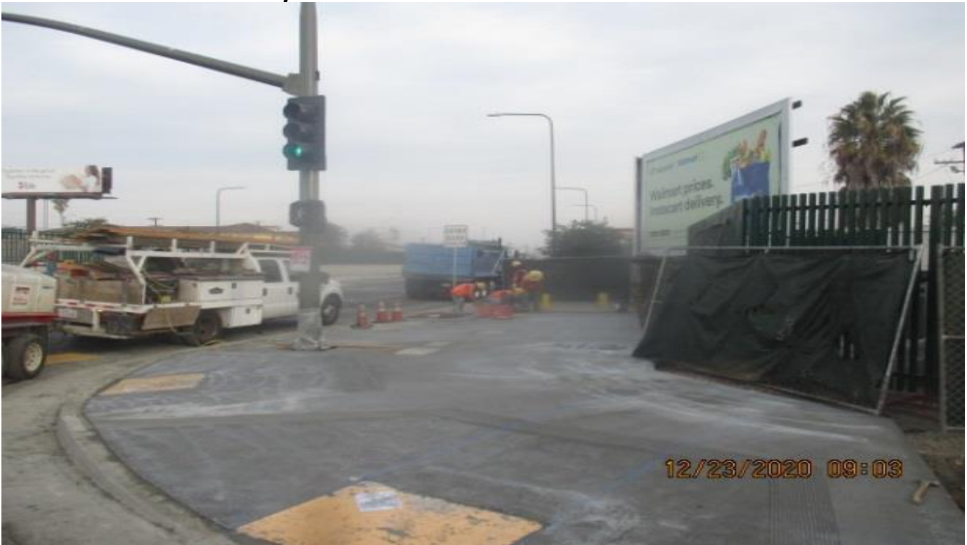
PARK MESA – Saw cut new sidewalk and ADA ramp and performed general clean-up on the northwest corner of 60th St and Crenshaw Blvd.
