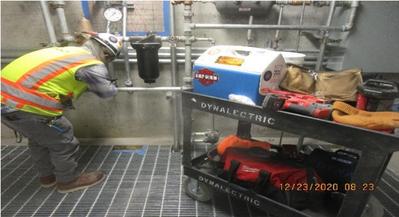
UG3 – Vernon Concourse, Ejector room C134, resume pipping 1” GRC (SCADA) between pump & control panel.
