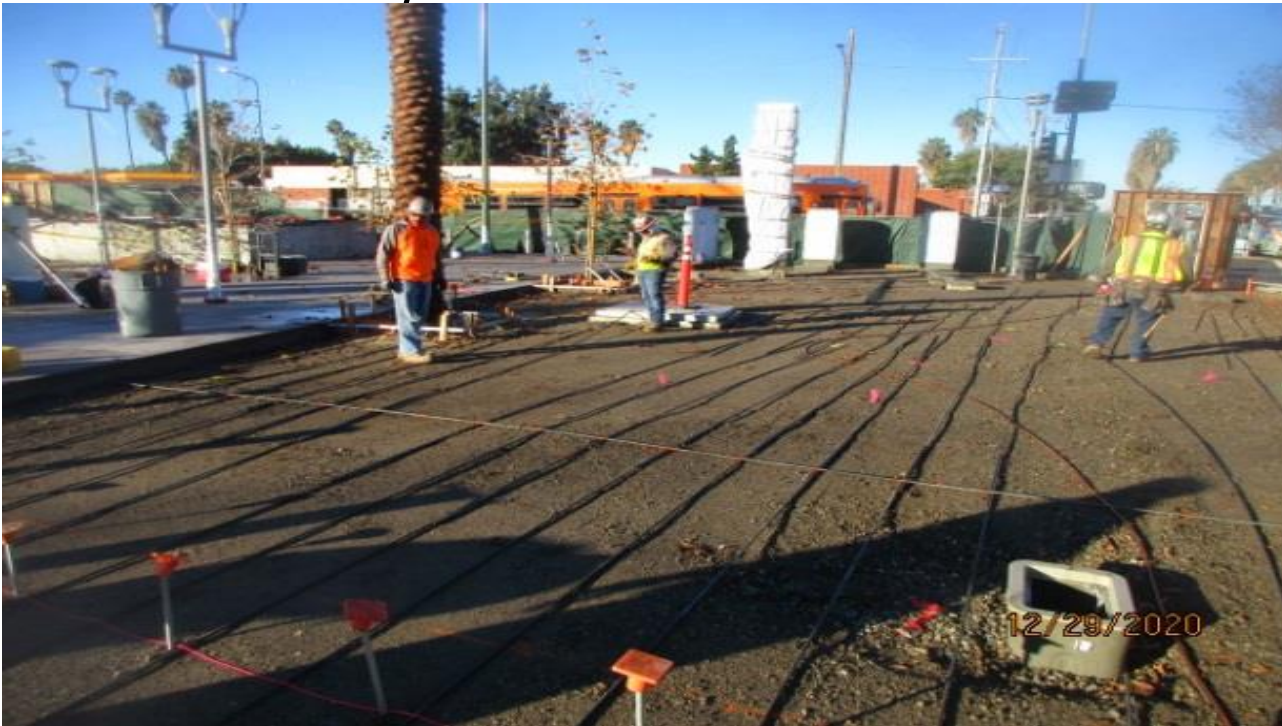
EXPO STATION – Continue building formwork and installing rebar for the architectural topping slab at the north side of the plaza.
