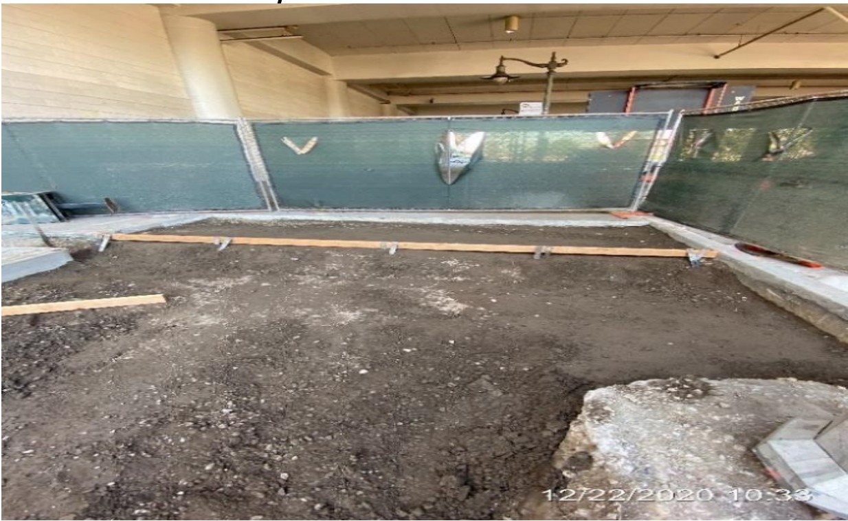
MLK STATION – Placing formwork for new sidewalk installation at the far northwest area of the plaza.
