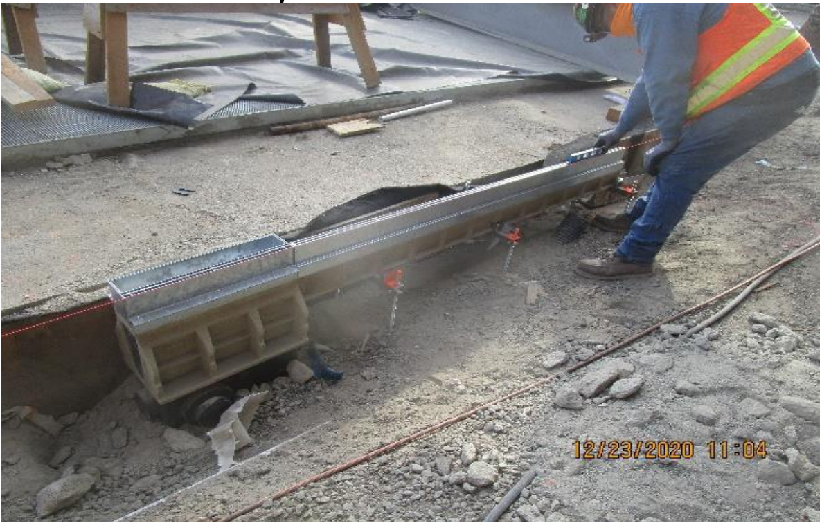
MLK STATION – ACO trench drains K100 type K 4” grate type 470 minimum fall not achieved due to design flaw.
