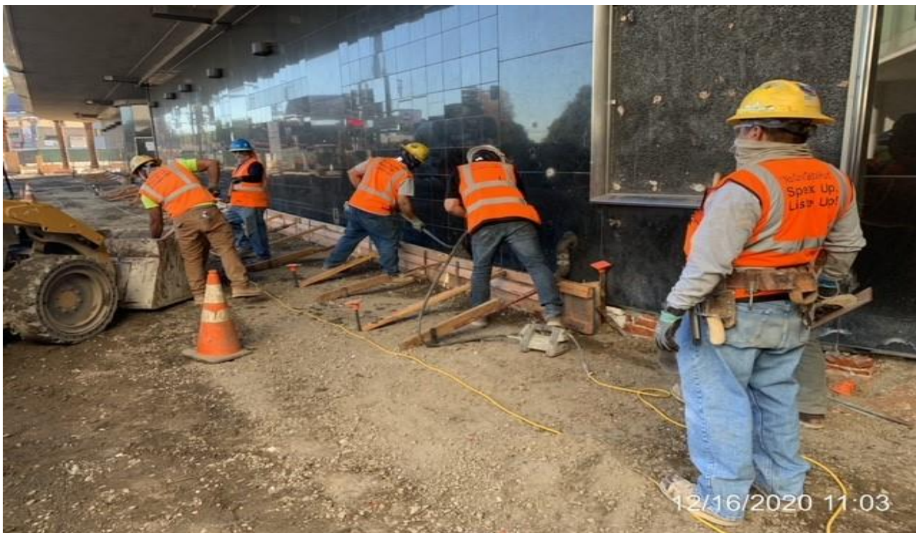
MLK STATION – WSCC crew placing concrete for short curb wall along north mall wall.
