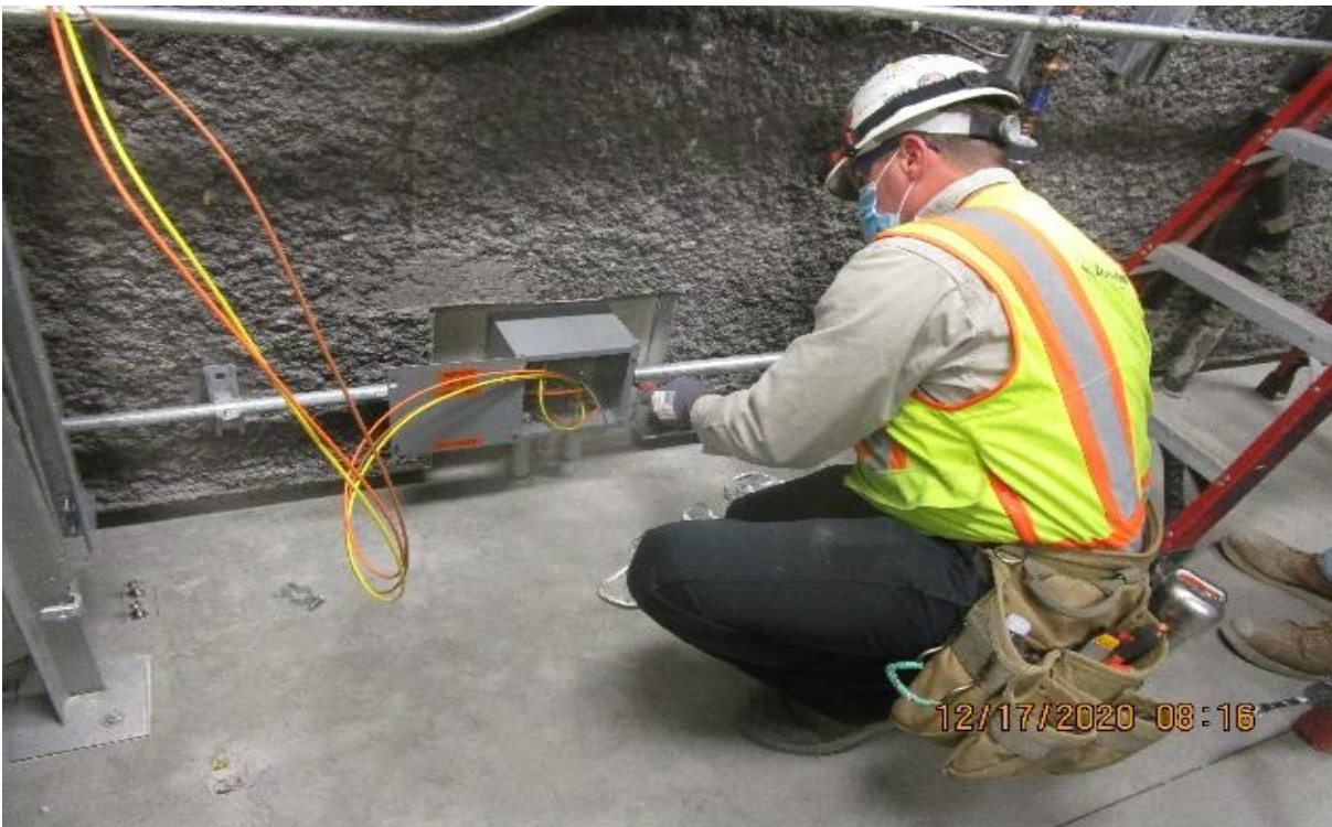
UG3 – Vernon, Mechanical room (N) C135, pipping 1” GRC to PAC-ACCP-2 control panel transformer cabinet
