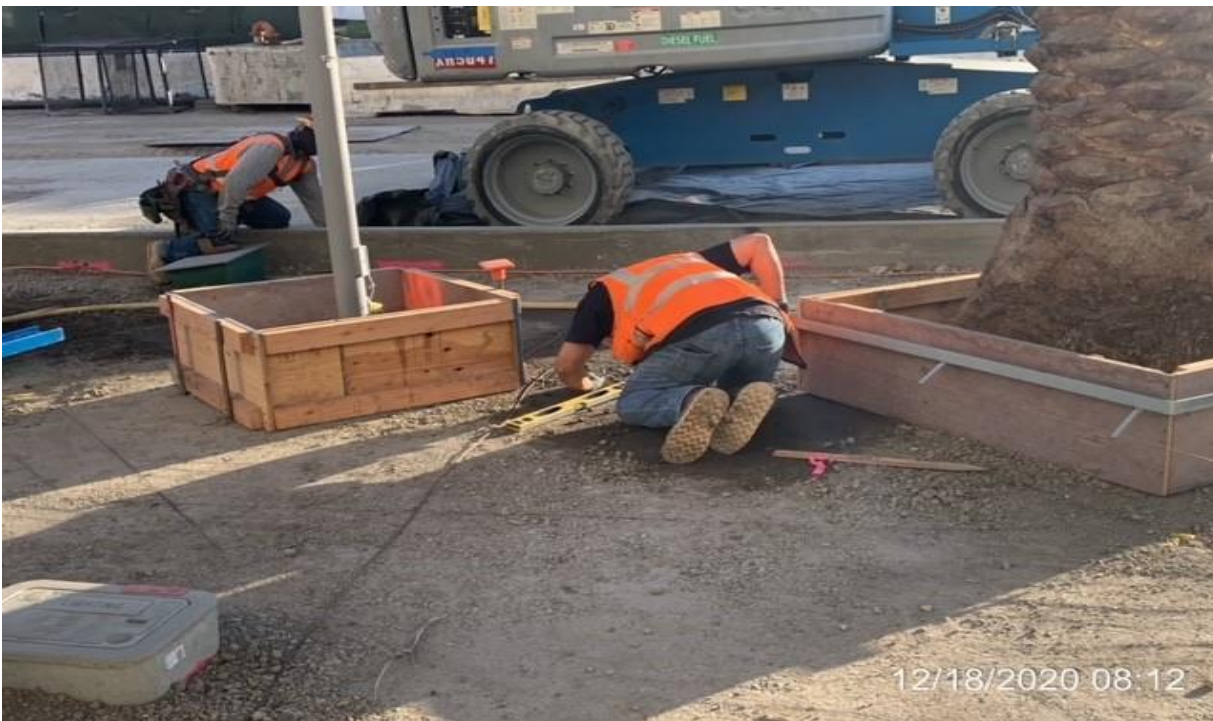
MLK STATION – WSCC carpenters at plaza level setting height for metal tree bases.
