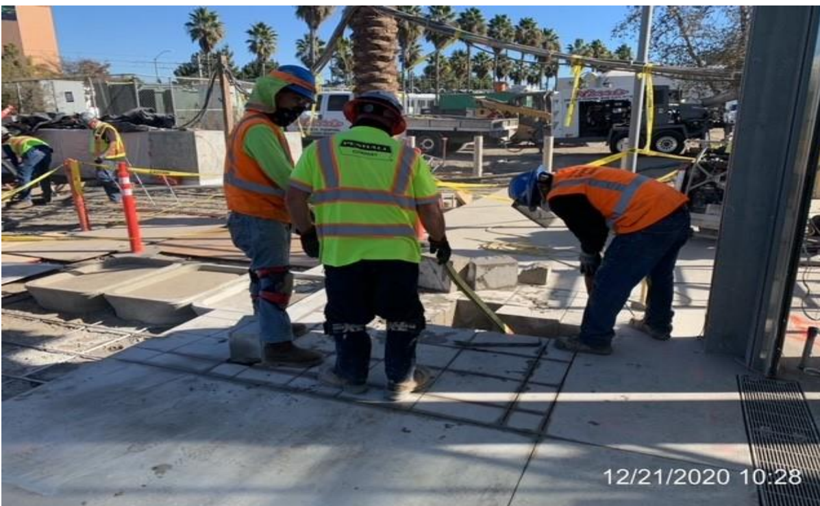
EXPO STATION – Penhall with WSCC laborers removing section of concrete slab to expose conduit.
