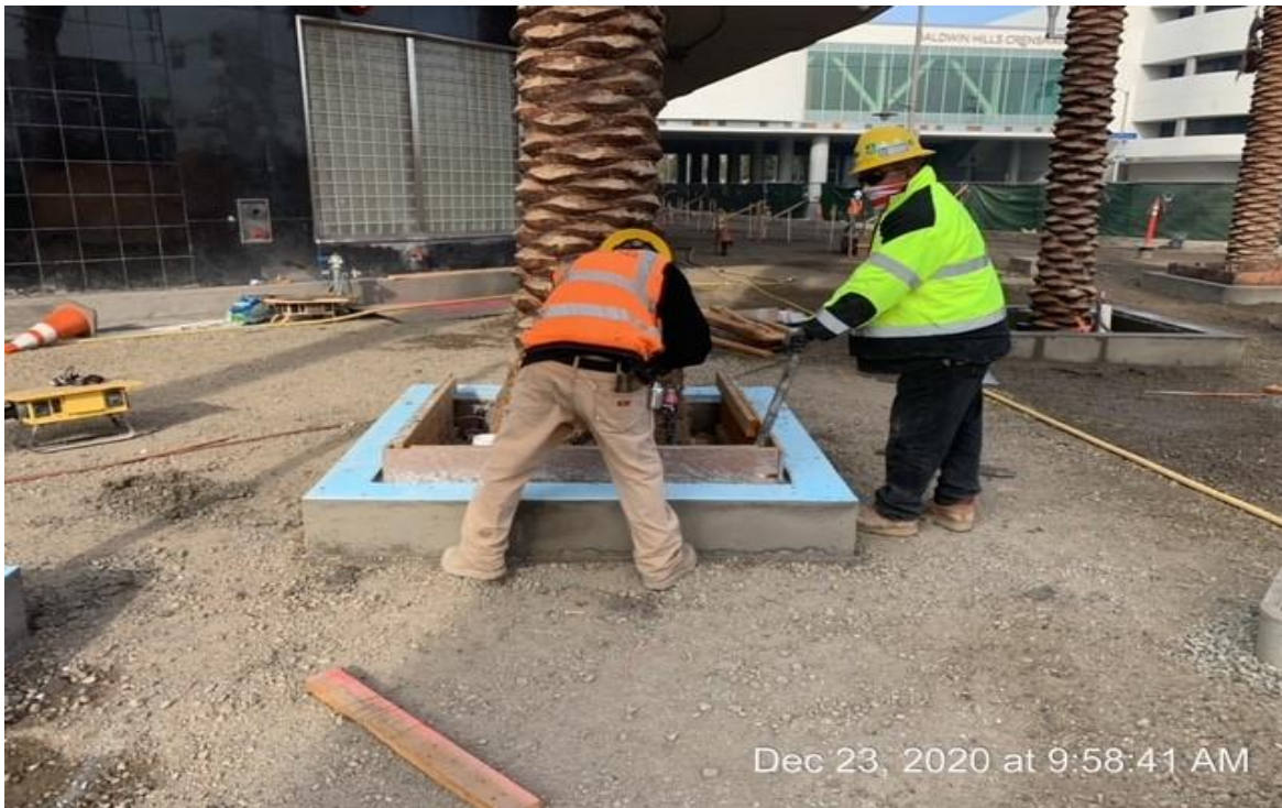
MLK STATION – WSCC crew removing formwork from tree and pedestrian light bases.
