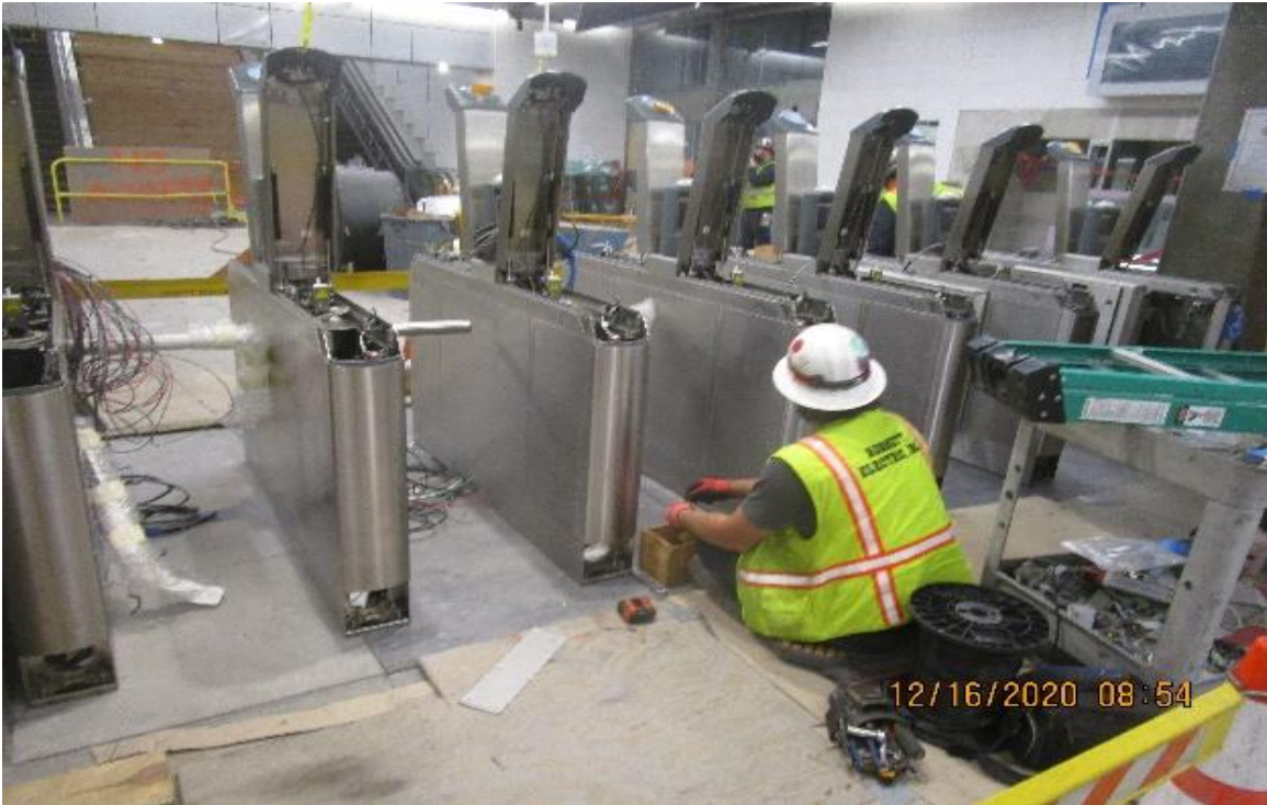
UG3 – Vernon, between Free Area C129 & Paid area C146 begin leveling & anchoring universal fare gate turnstiles.
