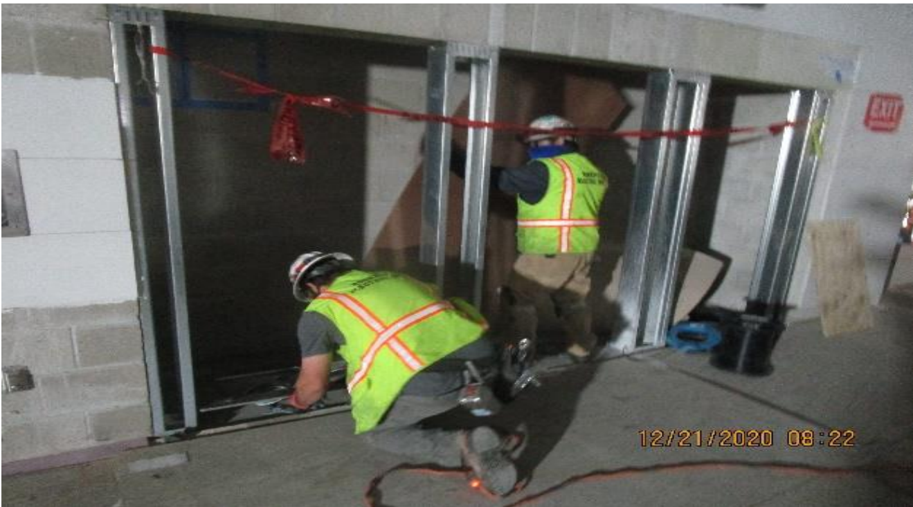
LEIMERT PARK STATION – Performing layout and coring for ticket vending machine installation at the Free Area..
