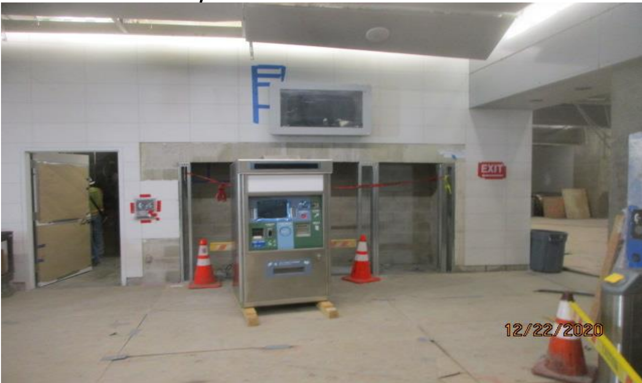
LEIMERT PARK STATION – Mobilizing and preparing for ticket vending machine installation at the Free Area.
