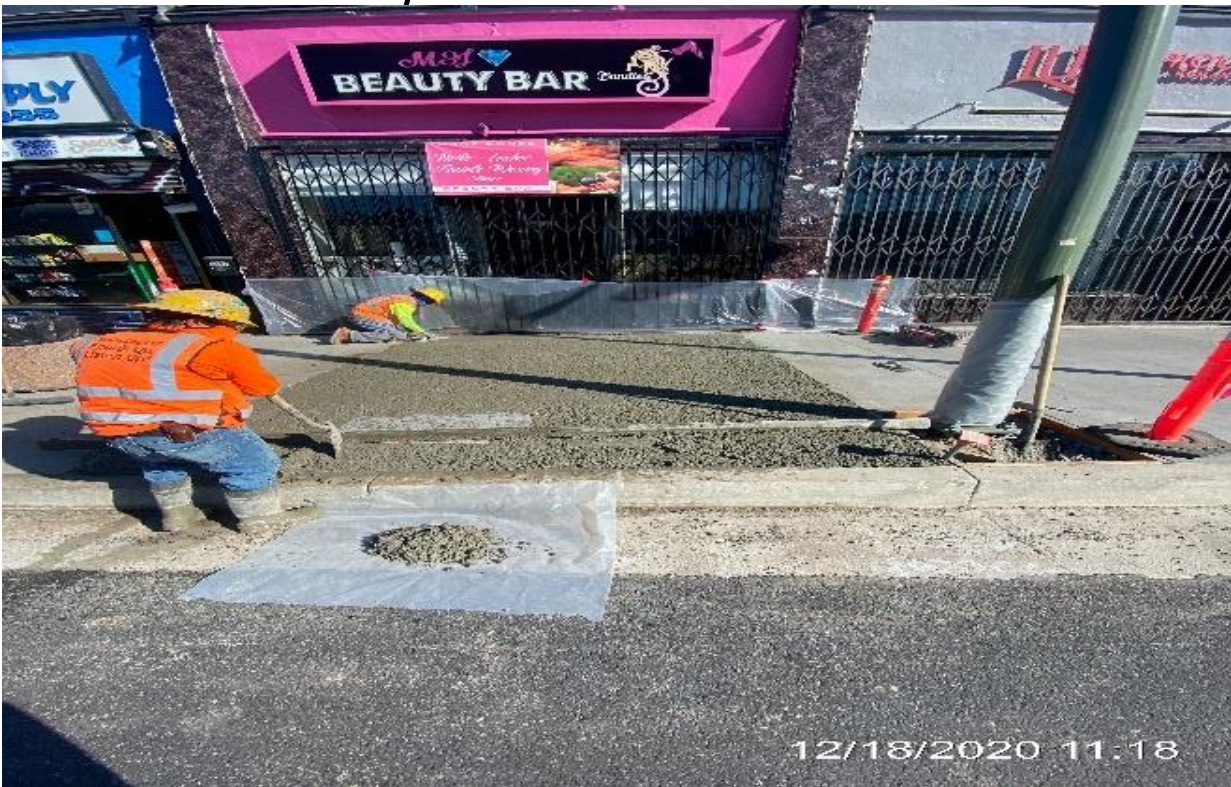
LEIMERT PARK STATION – Placed concrete for sidewalk section along northbound Crenshaw Blvd between 43rd Pl and Homeland Dr.
