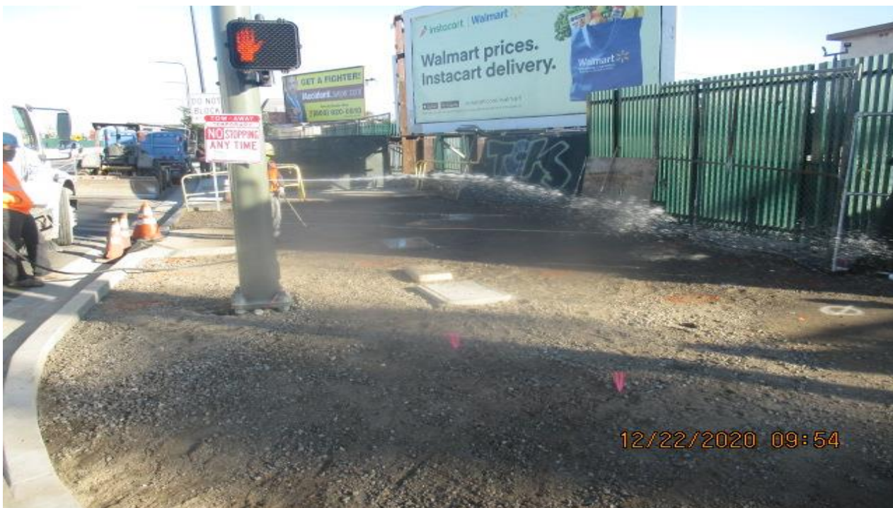
PARK MESA – Continue grading for new sidewalk and ADA ramp installation on the northwest corner of 60th St and Crenshaw Blvd.
