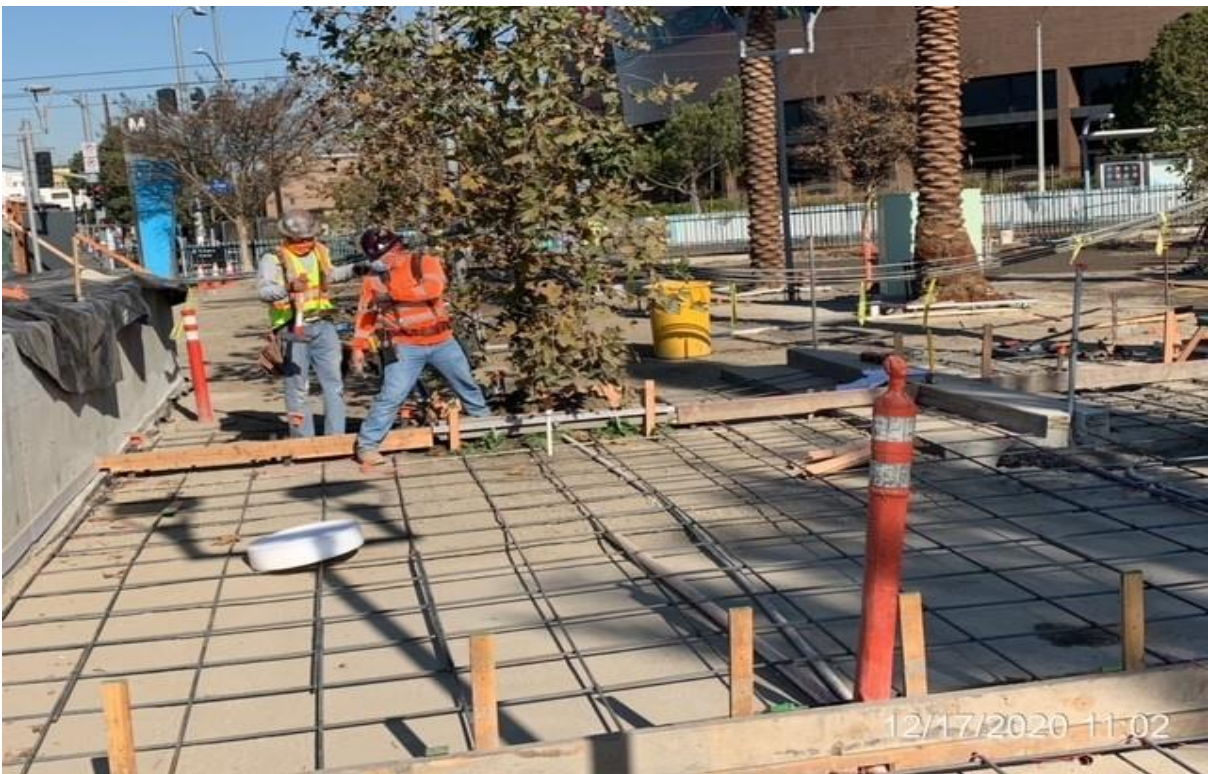
EXPO STATION – Dean Visosky installing formwork and #4 rebar for slab at sec 12 and 13.
