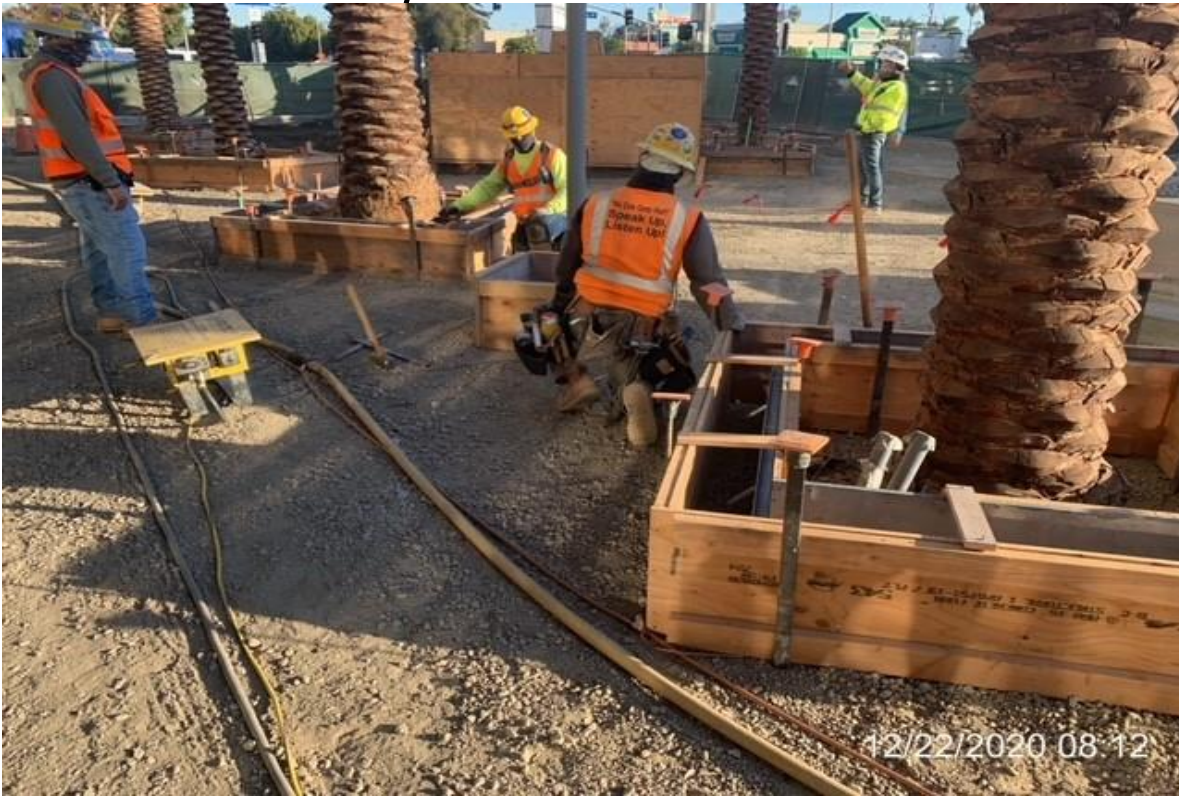
MLK STATION – WSCC carpenters setting formwork for tree and pedestrian light bases.
