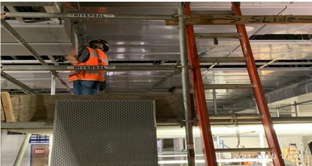
EXPO STATION – Installing ceiling panels above Escalator 3&4 at the Paid & Free Area.
