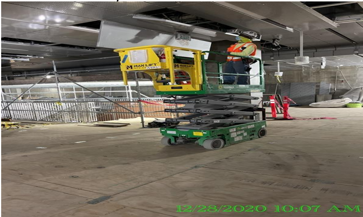
EXPO STATION – Installing LED light fixtures to the drop ceiling of the Paid & Free Area.
