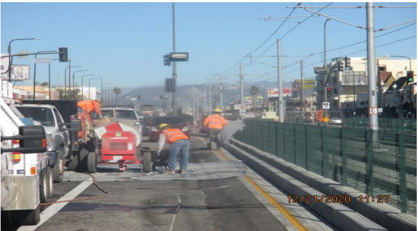
PARK MESA – Mixing and placing mortar base for cobble placement on the southbound median from Slauson Ave to 57th St.
