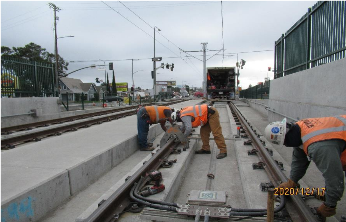
PARK MESA – HCC removing DF fasteners visually inspecting concrete bonding to inserts on SB track near 48th Street (looking south)
