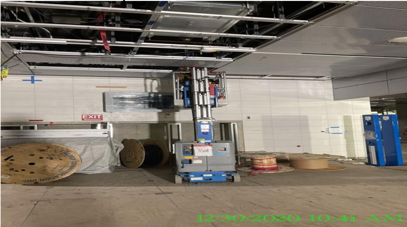
EXPO STATION – Continue installing LED light fixtures to the drop ceiling of the Paid & Free Area.
