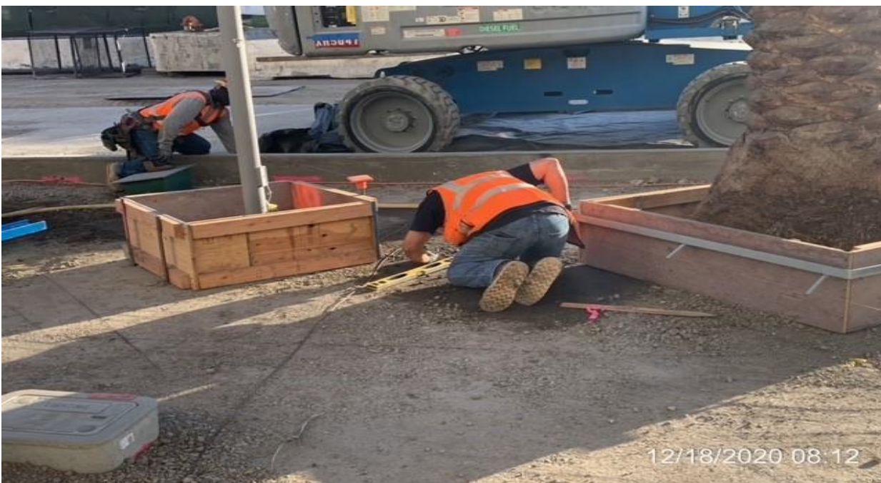
MLK STATION – Setting metal frame heights for palm tree bases at the plaza.
