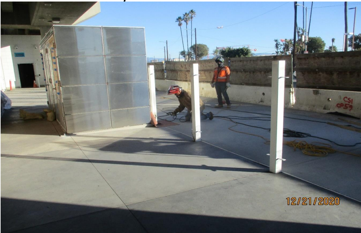
AVIATION/CENTURY- Rewelding the flanges to the fence post at the Aviation Station.
