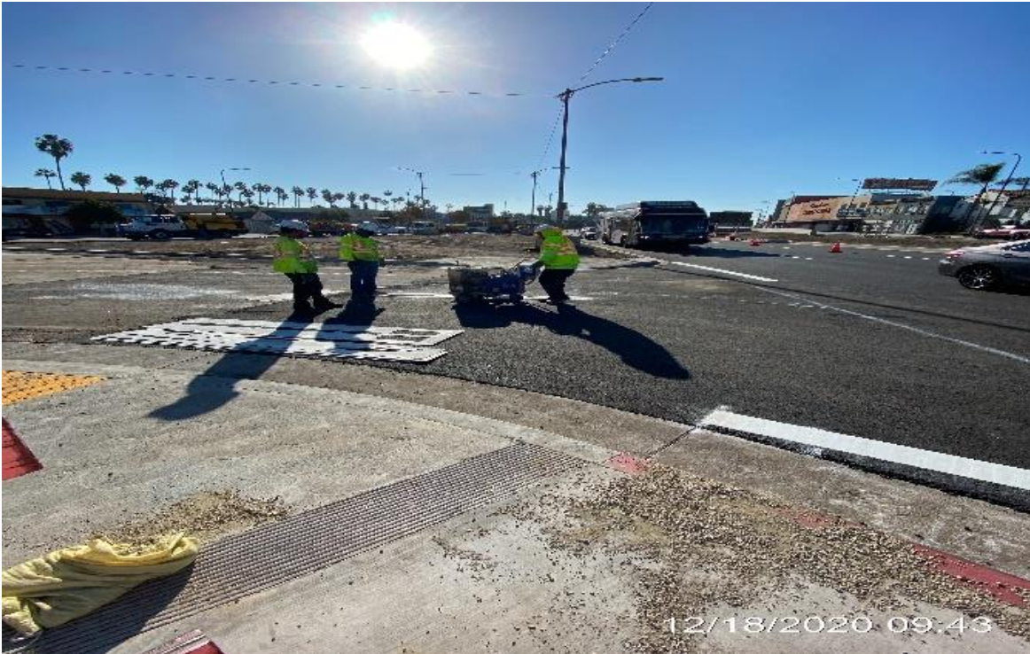
PARK MESA – Continue installing guardrails along the north and southbound side of the south end entrance ramp.
