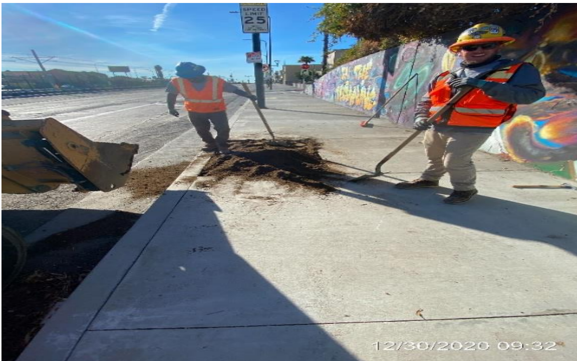
PARK MESA – Continue placing top soil to tree wells along southbound Crenshaw Blvd between 52nd St. and 50th St.
