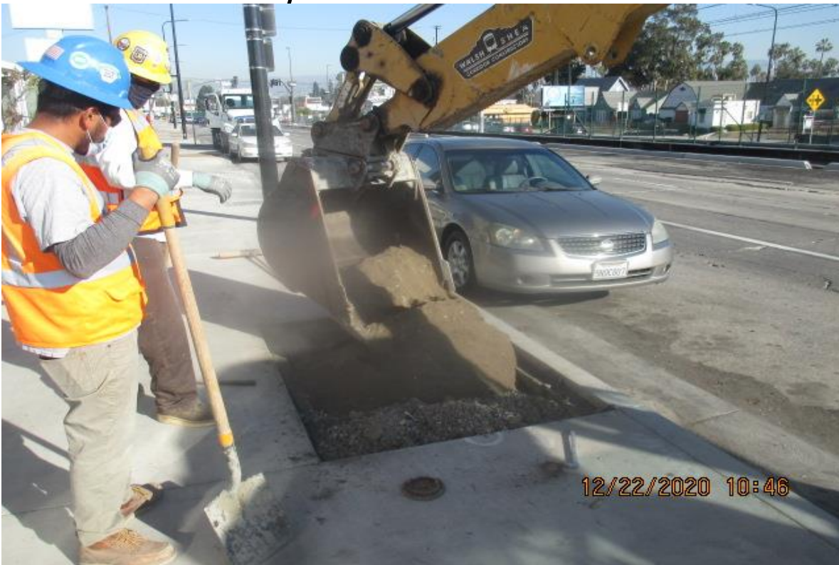
PARK MESA – Placing top soil to tree wells along southbound Crenshaw Blvd between 50th St. and 48th St.
