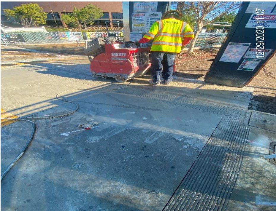
EXPO STATION – Saw cutting control joints for new sidewalk and ADA ramp on the northwest corner of the plaza.
