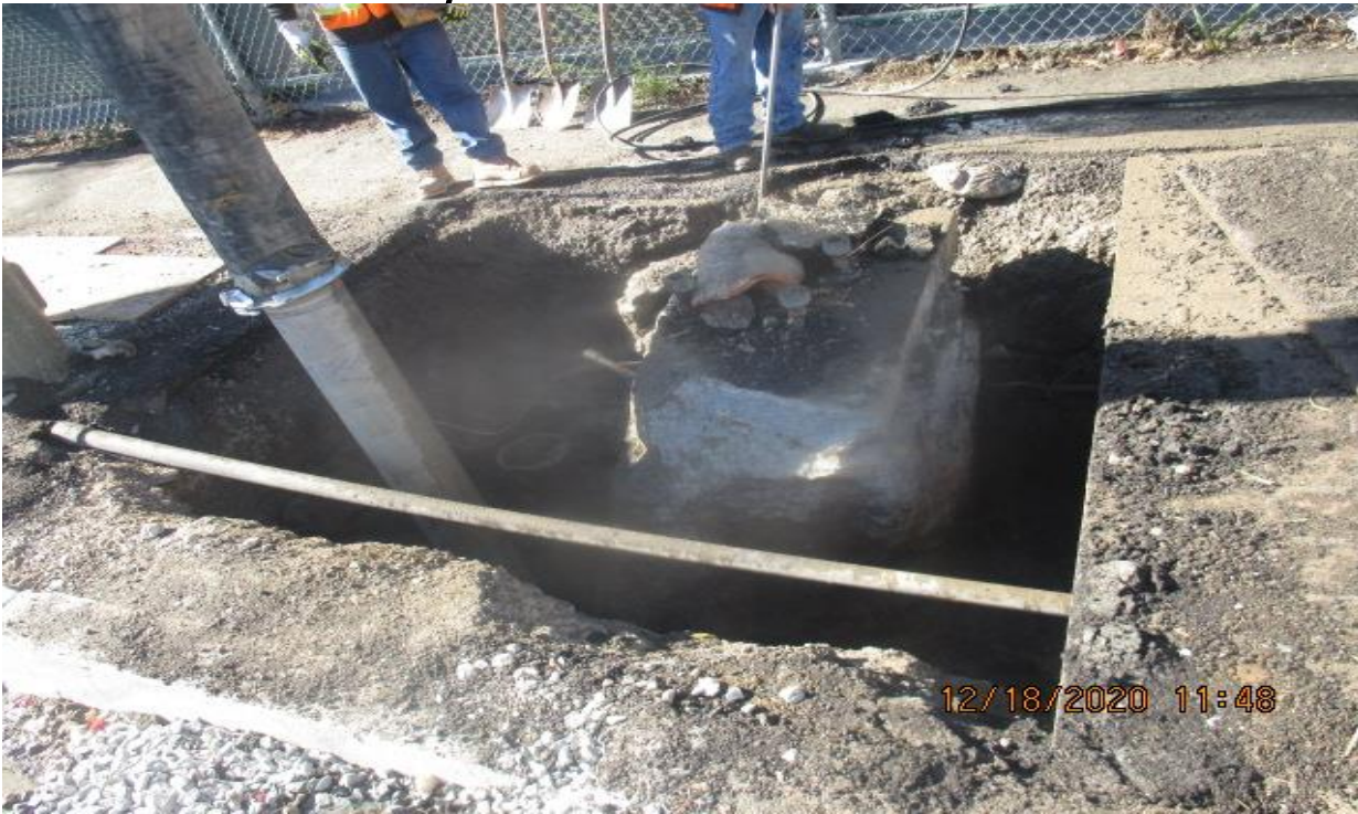
PARK MESA – Removing existing street light foundation on the southwest corner of 60th St and Crenshaw Blvd.
