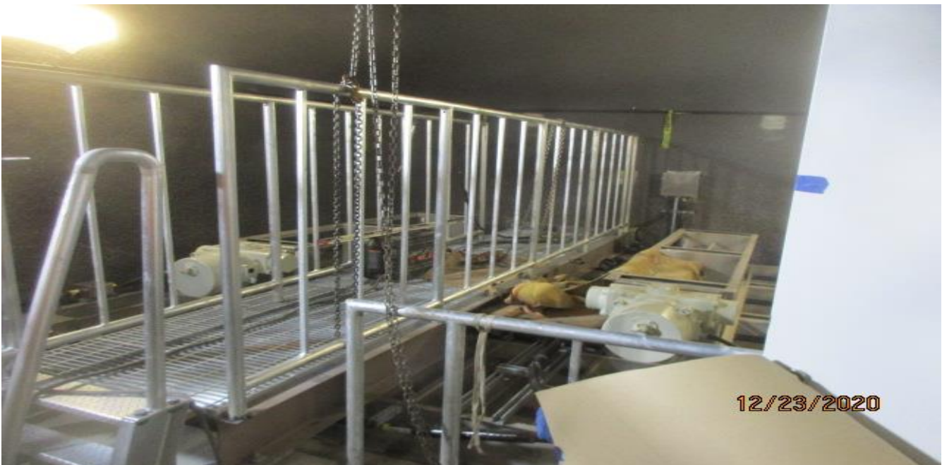
LEIMERT PARK STATION – Continue drilling and installing guardrails around the dampers inside the Emergency Ventilation Shaft/OTE Plenum North C-127 and South C-101.
