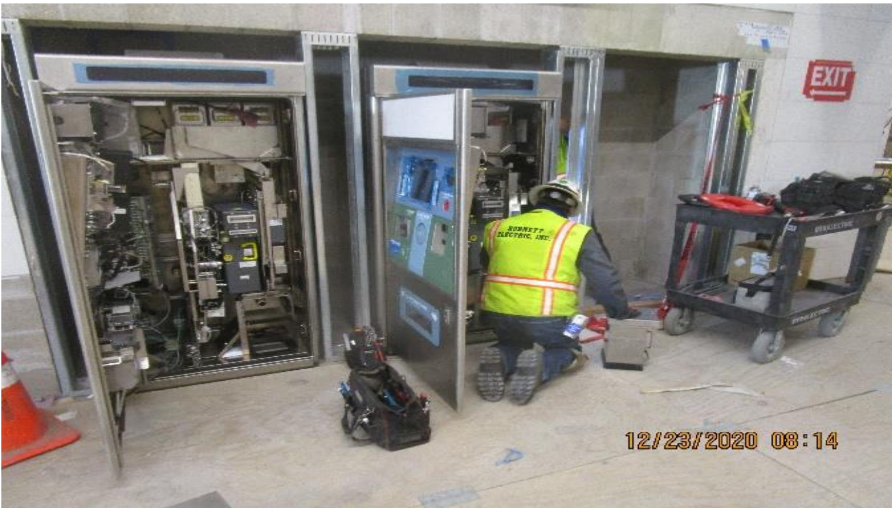
LEIMERT PARK STATION – Continue installing and wiring the ticket vending machines at the Free Area.
