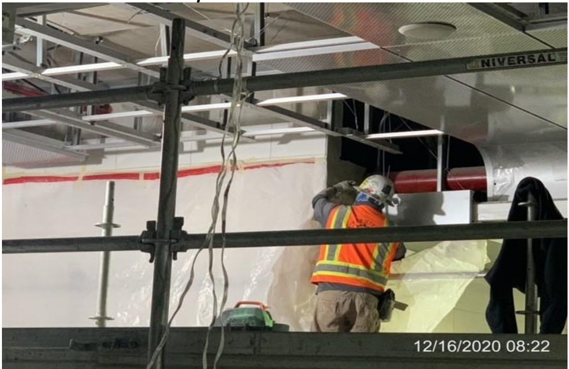
EXPO STATION – Premier Tile & Marble removing tile from above stair #2 and escalator #3.
