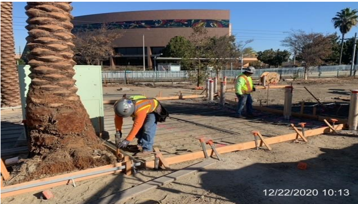
EXPO STATION– Continue building formwork and installing rebar for the architectural topping slab at the north side of the plaza.
