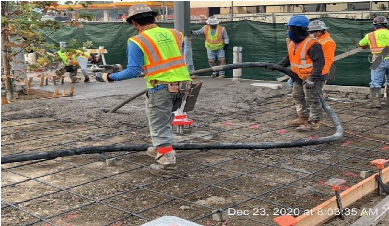
EXPO STATION– Continue placing concrete for the architectural topping slab at the north side of the plaza.
