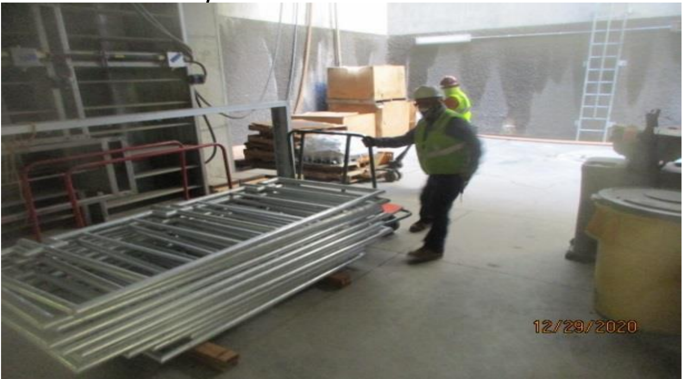
MLK STATION – Mobilizing material for guardrail installation around the dampers inside the Emergency Ventilation Shaft/OTE Plenum North C-143 and South C-101.
