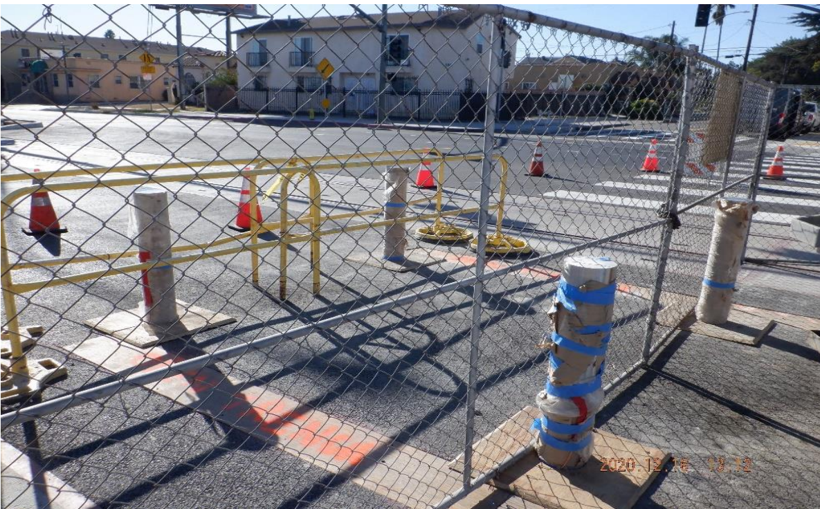
PARK MESA – STA 317+50 TK#4/NB looking west – 59th St at grade crossing – new bollards set-up in the crosswalk between tracks.
