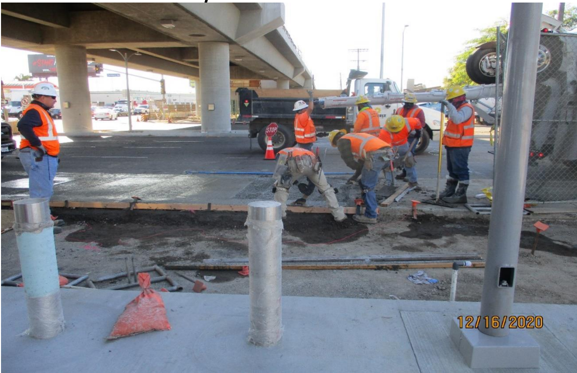
AVIATION/CENTURY- Placing concrete for the sidewalk on the NW corner of Aviation and Century.
