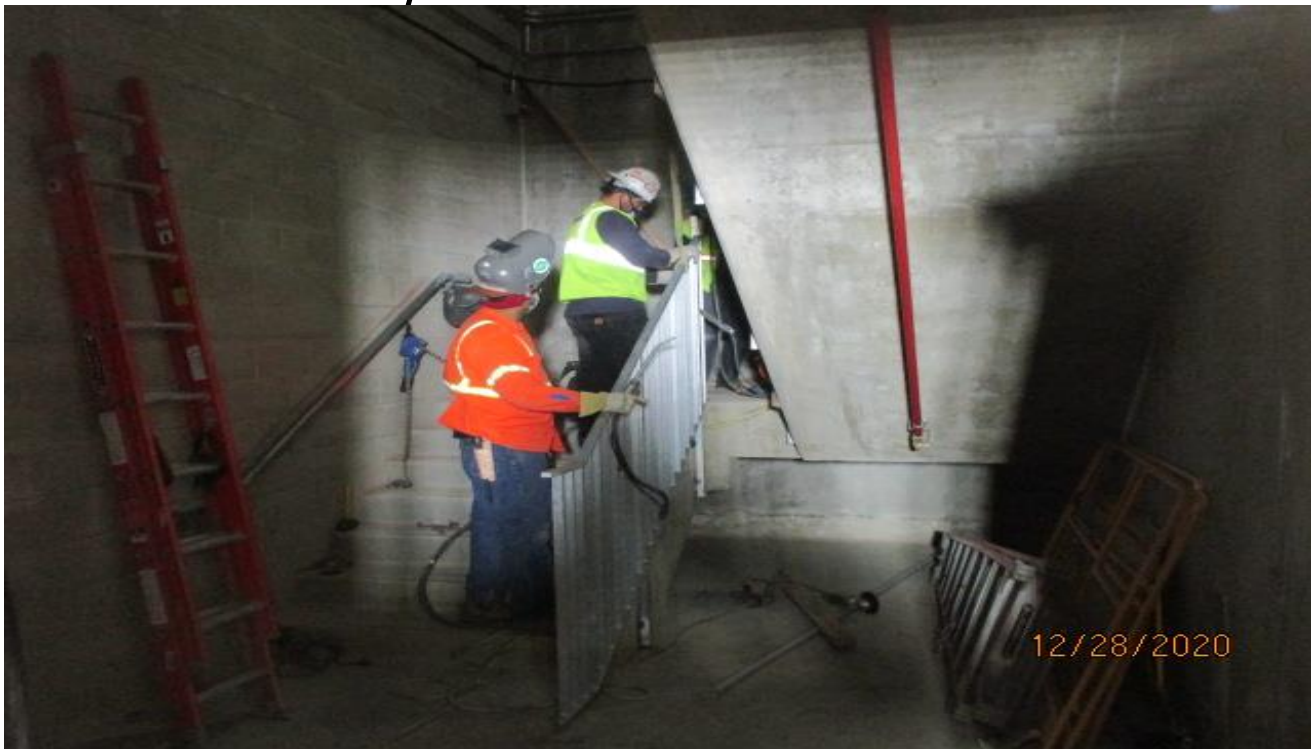
EXPO STATION – Resume guardrail installation of Emergency Exit Stair 3 at the invert level.
