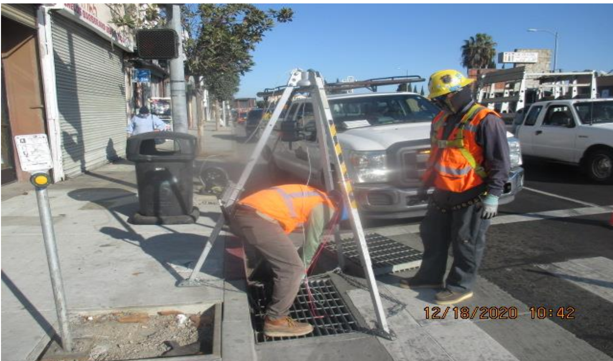
PARK MESA – Installing grates to Catch Basin #2 on the northwest corner of Hyde Park Blvd and Crenshaw Blvd.
