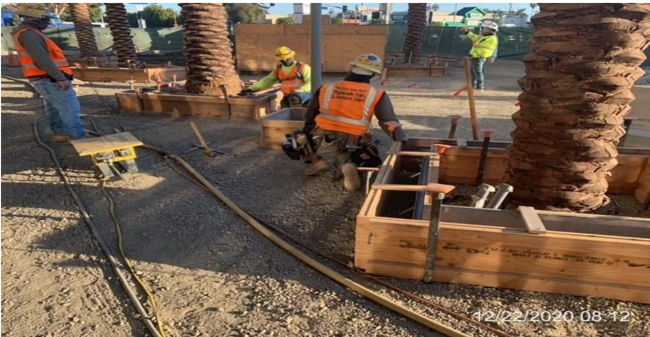
MLK STATION – Continue setting formwork for palm tree and pedestrian light pole bases at the plaza.
