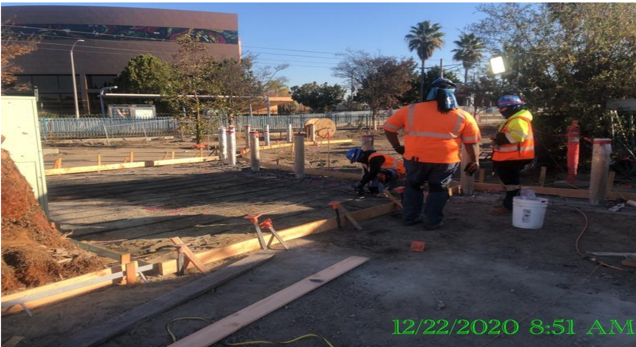
EXPO STATION – Continue ground grid installation at the north side of the plaza.
