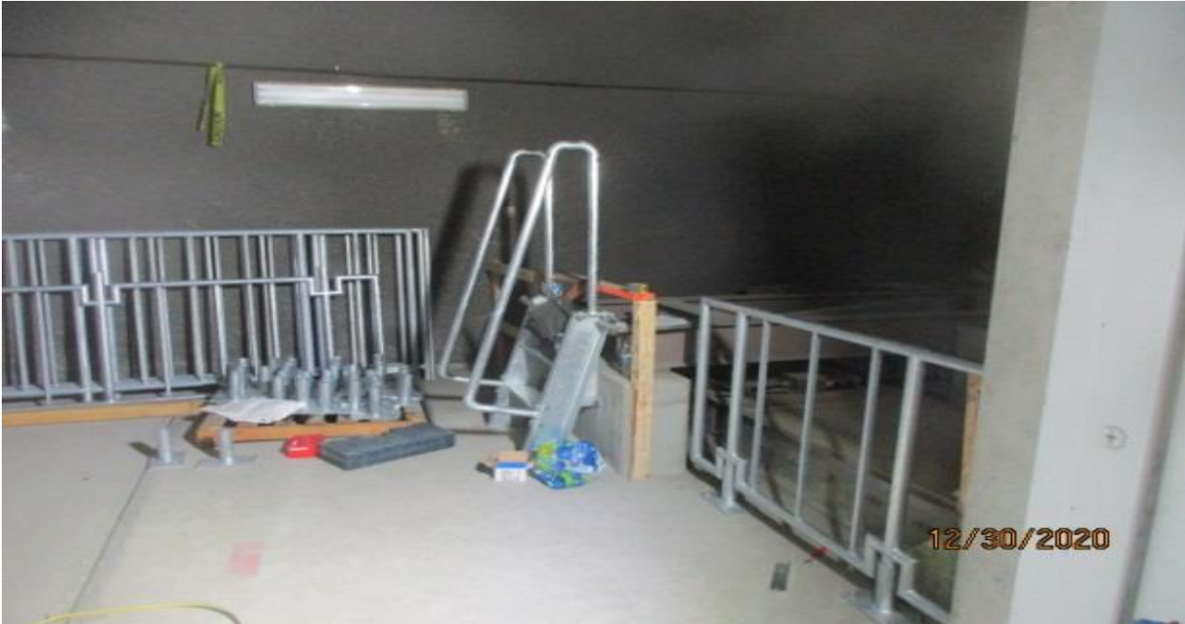
MLK STATION – Installing guardrails around the dampers inside the Emergency Ventilation Shaft/OTE Plenum South C-101.
