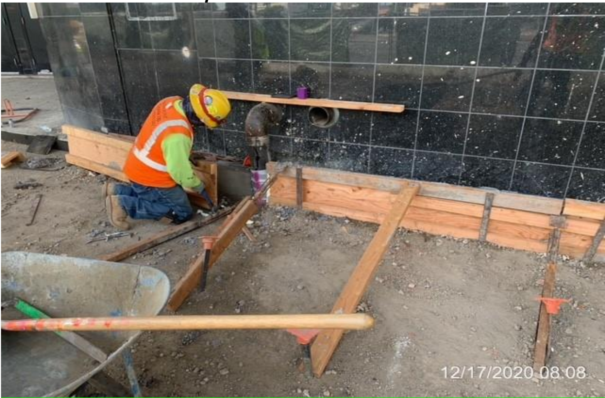
MLK STATION – WSCC crew removing forms from short curb wall along north mall wall.
