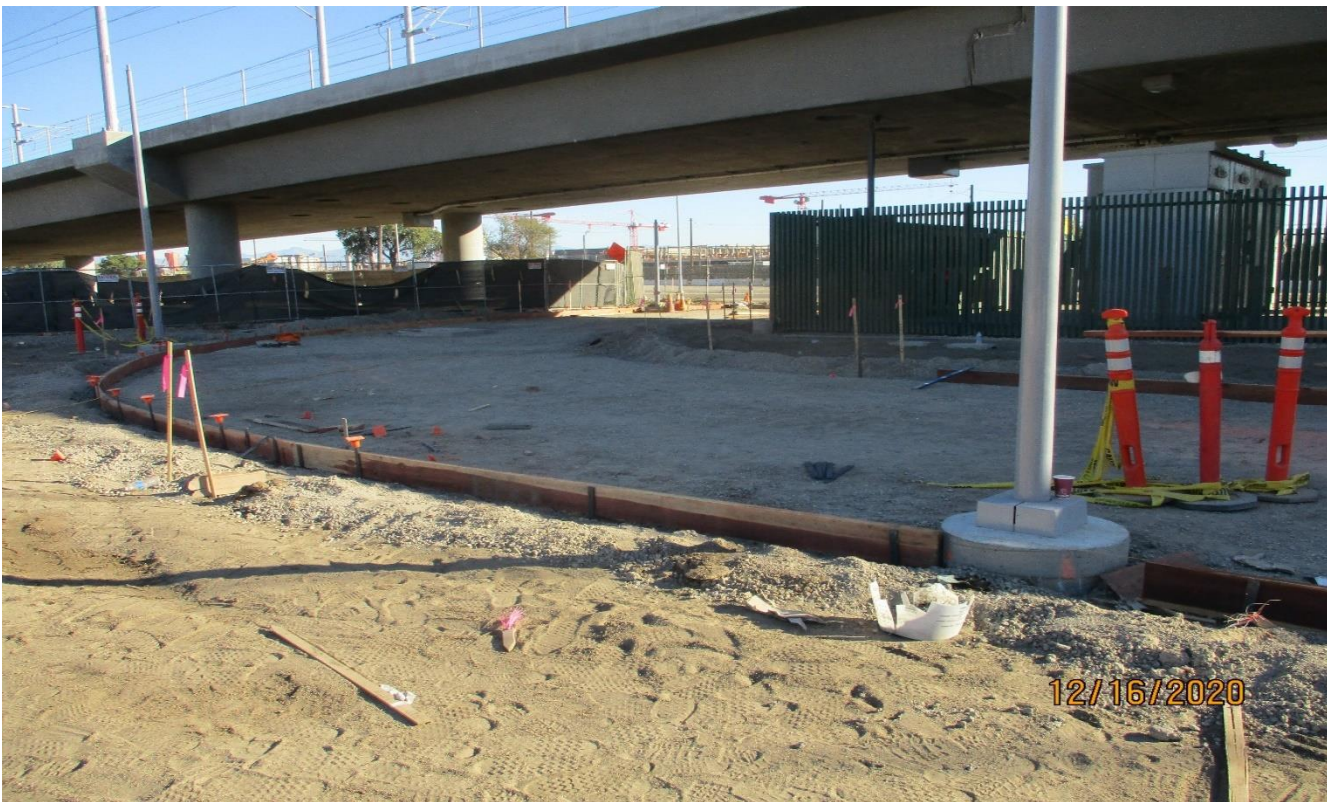
AVIATION/CENTURY- Setting header boards for the service driveway at the Aviation Station.
