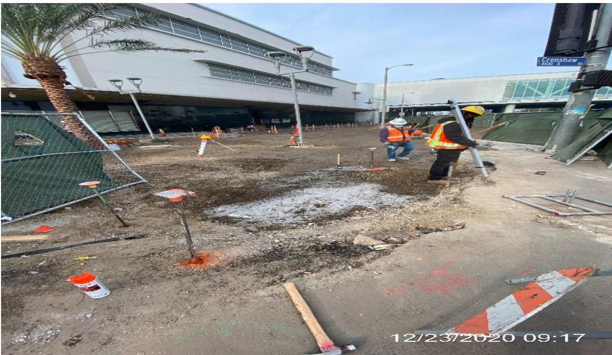
MLK STATION – Setting elevations for new sidewalk and ADA ramp installation on the northeast corner of the plaza.
