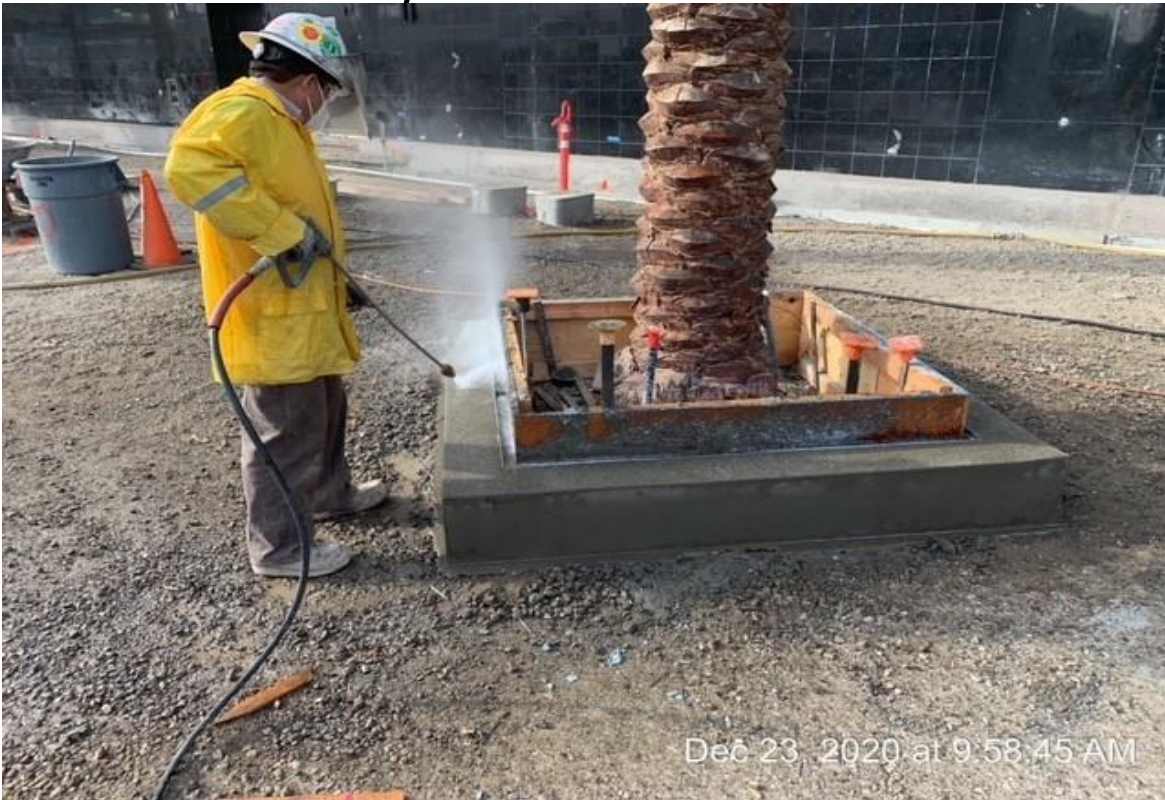
MLK STATION – WSCC finisher removing top cast paste from tree and pedestrian light bases.
