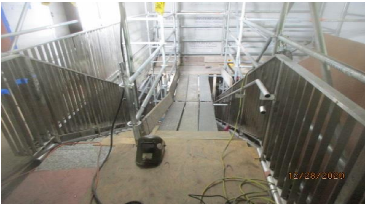
EXPO STATION SITE – Resume handrail installation to the guardrails of Staircase 2&3 from concourse to platform.
