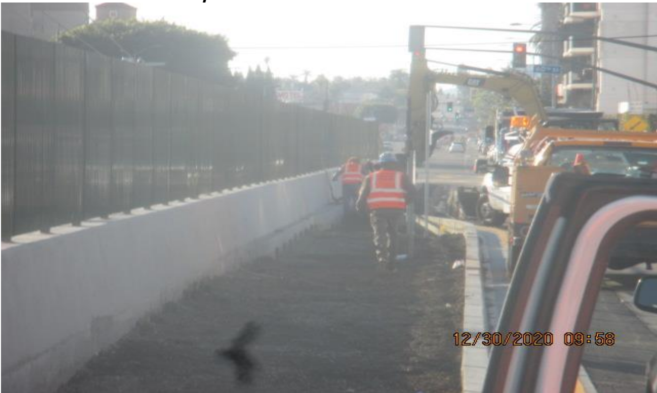
PARK MESA – Excavating/grading southbound median of Crenshaw Blvd from 60th St to 59th St.
