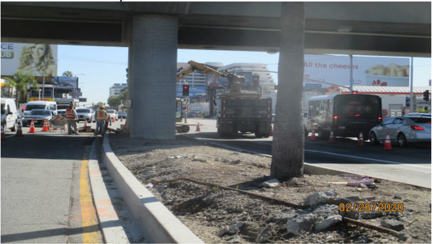
Aviation/Century – Demo of the median island bull nose at the west quadrant of the Century and Aviation intersection.
