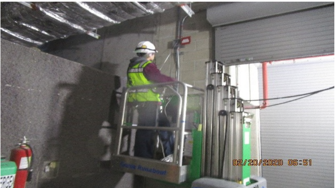
Crenshaw/Vernon - Tunnel vent plenum (S) 2 C106, begin pulling strobes (1) pair #14) to Equipment access (S) C107 devices.
