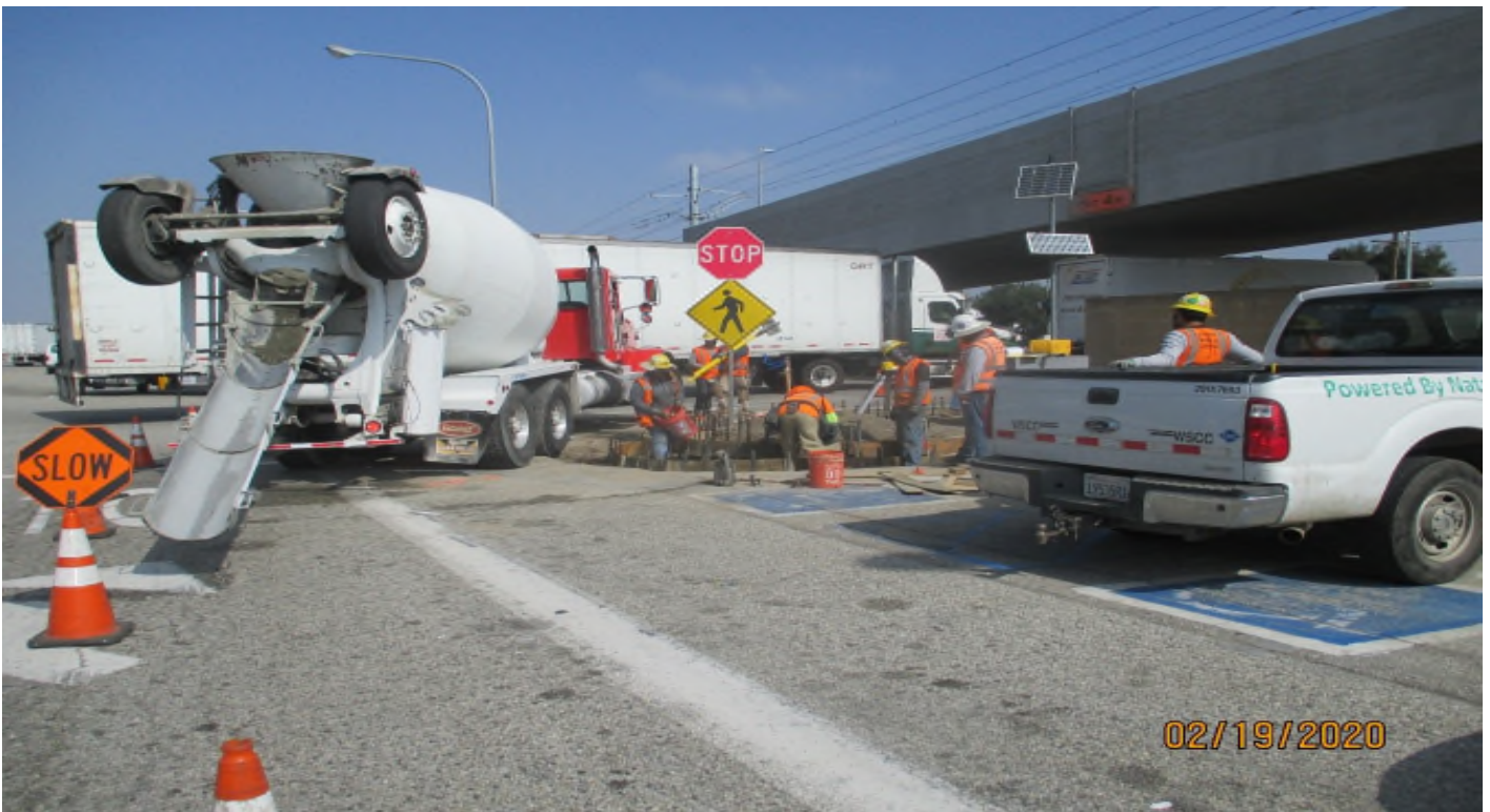
111 th Street – Start of the concrete placement on 111th street. Facing north.
