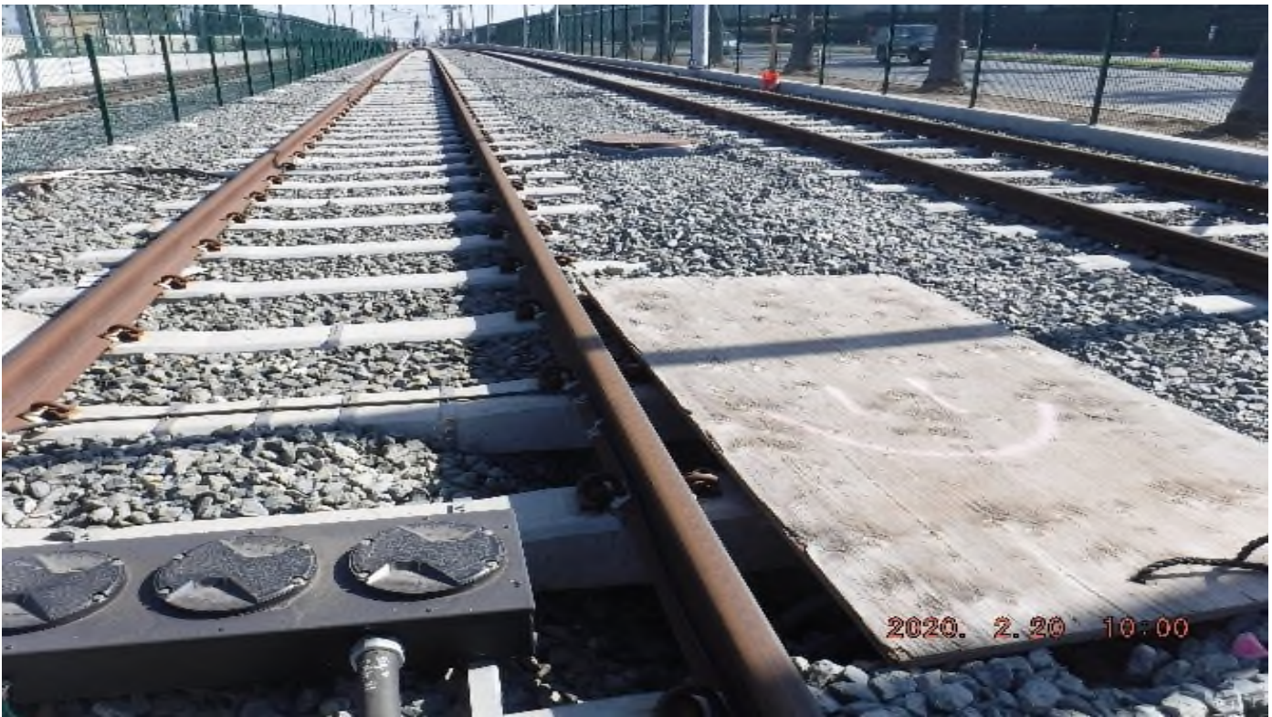
Centinela Ave. – STA 249+50 TK#3 SB looking north – disturbed track structure @ S461, S462.
