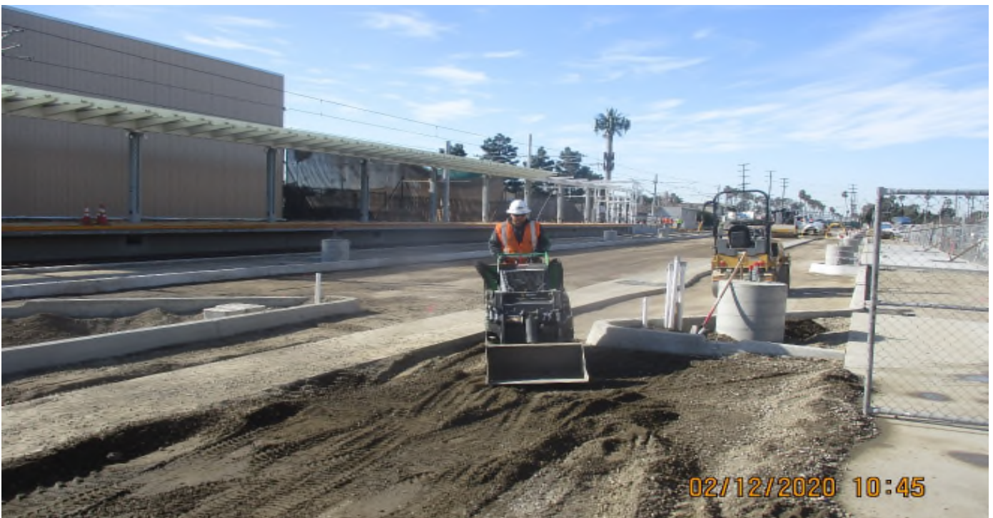
Florence/West – WSCC Making fine grade for asphalt at West Sta parking lot.
