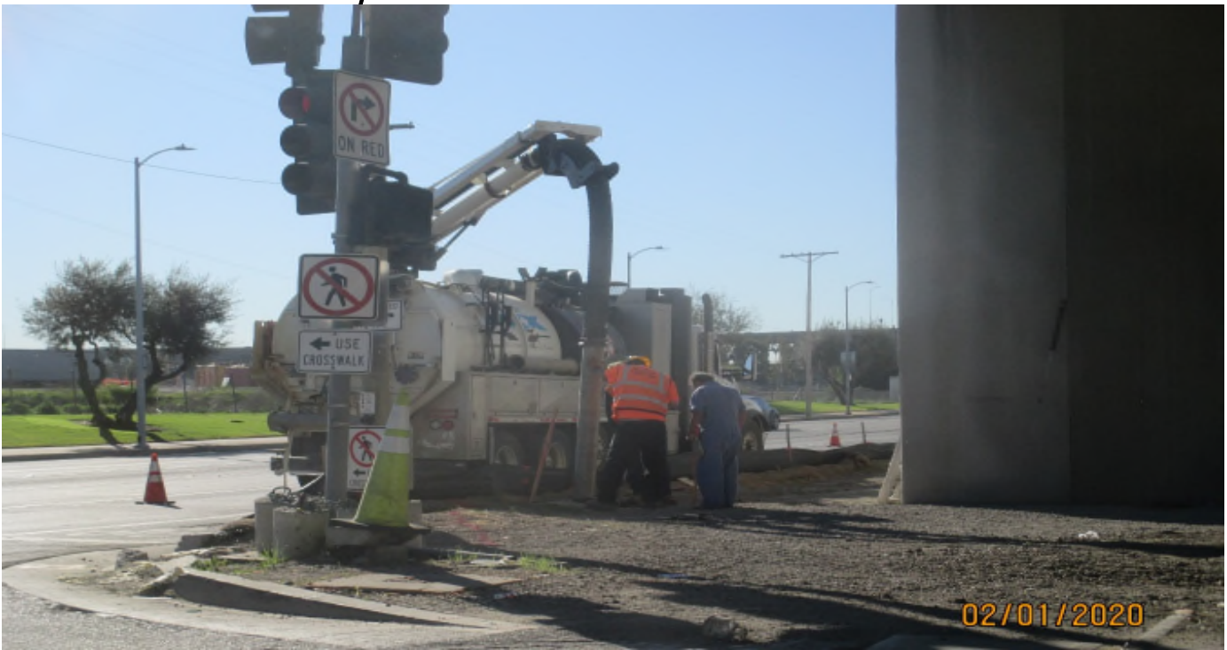
Aviation/Century – Vacuum truck exposing the gas line at the SW corner of 111th street and Aviation.
