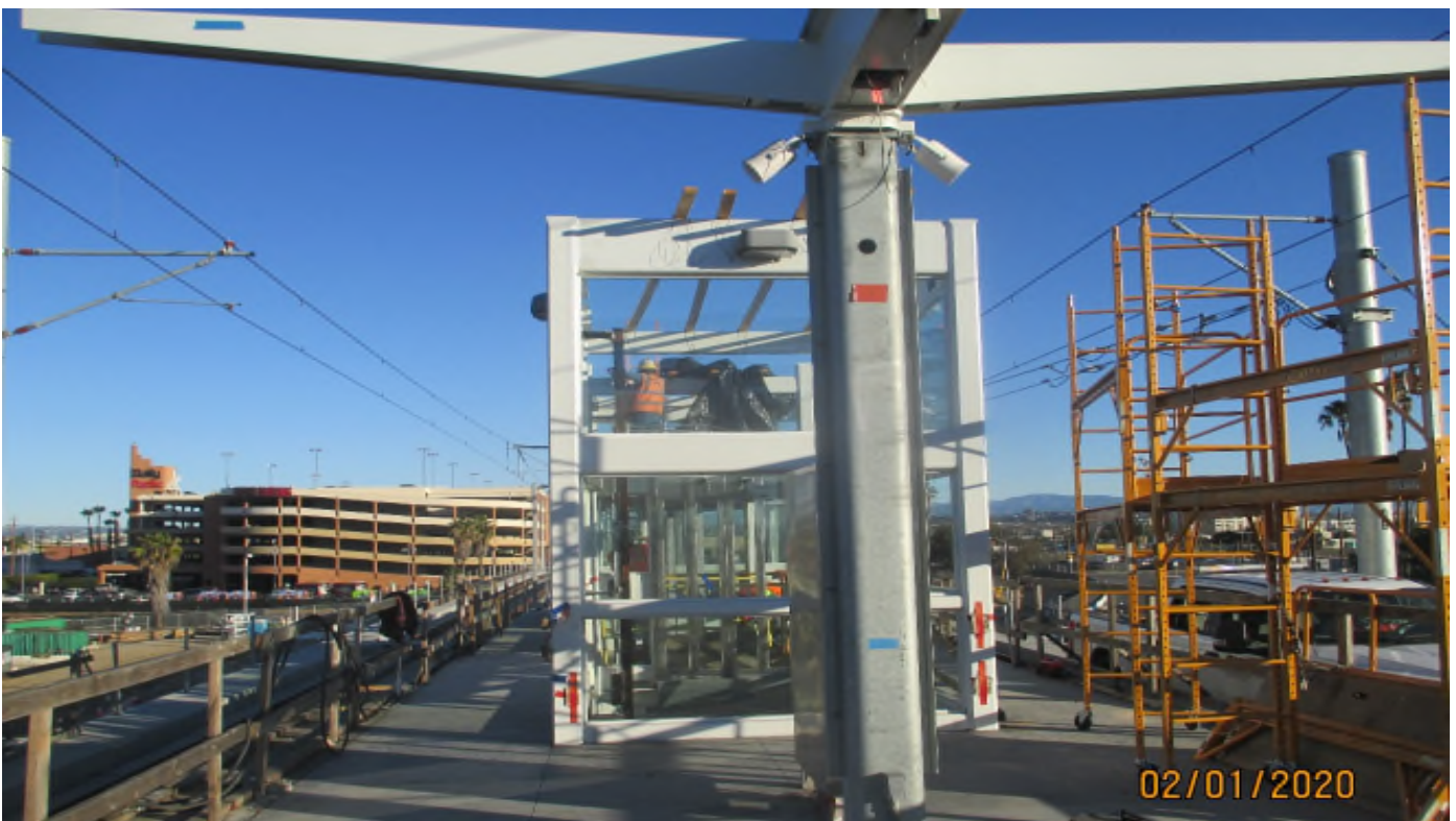
Aviation/Century – Removal of the rain cover and wood at the Aviation Station elevators.
