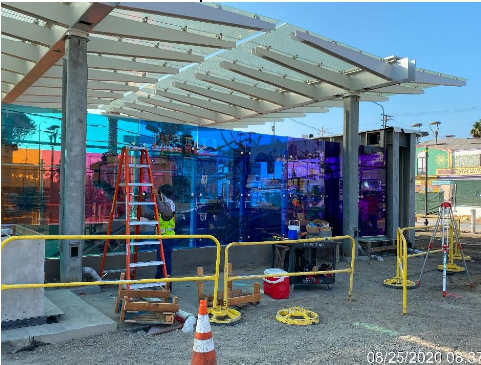
LEIMERT PARK STATION – Continue installing art glass panels around the main entrance canopy structure at the plaza level.
