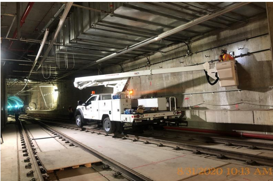
EXPO STATION – Continue installing supports and fixtures for the crossover lighting at the invert level.
