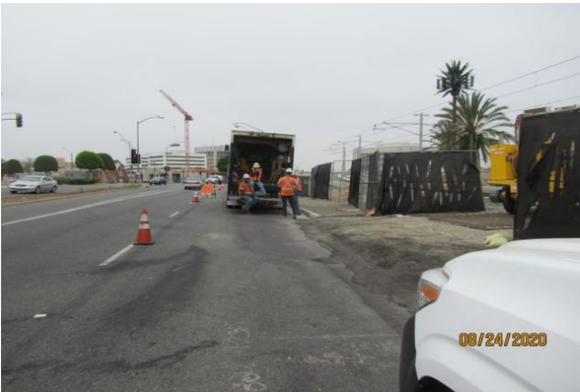
La Brea – HCC track gang at La Brea waiting for LKC to remove track wiring.
