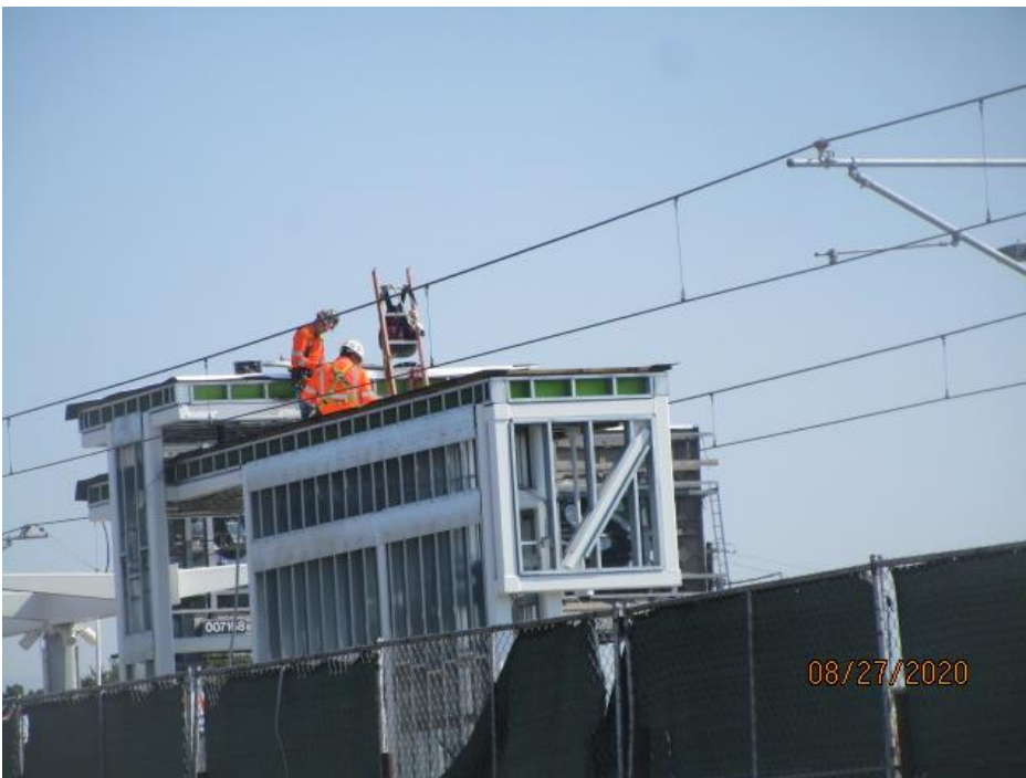
HYDE PARK STATION SITE – Continue installing roofing to the canopy on the south and north end of the platform level.
