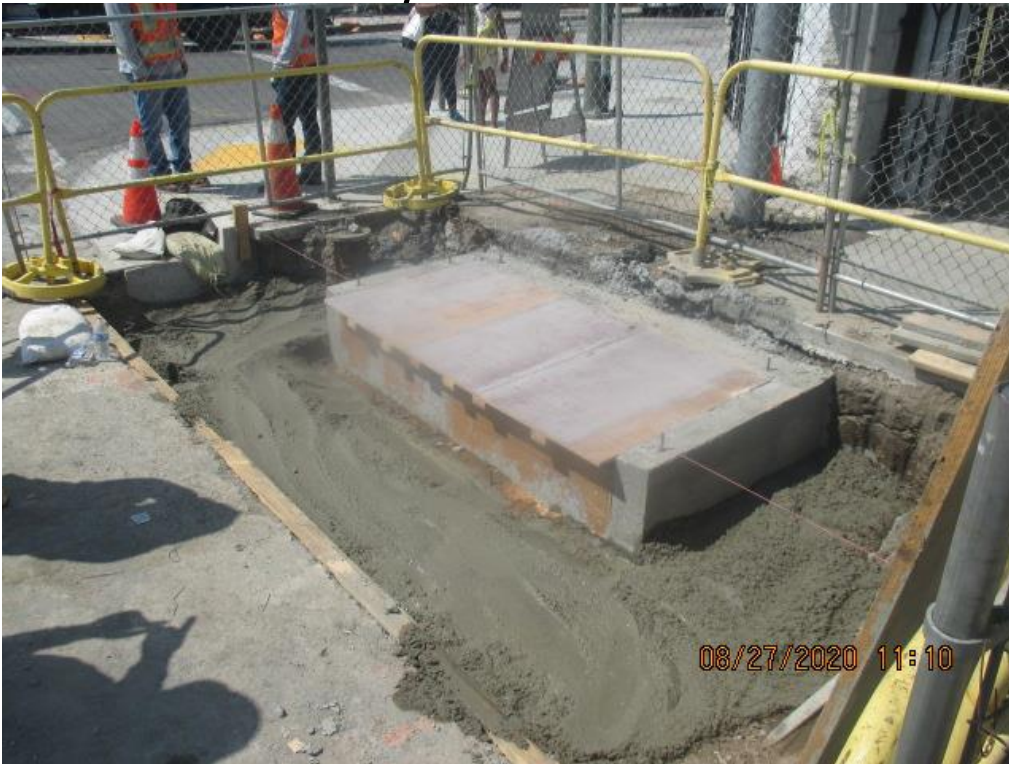
PARK MESA – Placing slurry backfill for Catch Basin #30 on the northeast corner of Crenshaw Blvd and 67th St.
