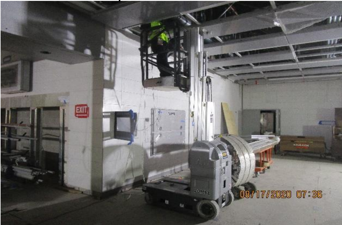
Crenshaw/Vernon – Vernon, Paid Area C146, pulling 1 pair 18 & 1 pair 14 from battery room C120 to FATC for smoke detector
