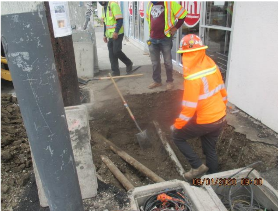
PARK MESA – Continue excavating for pull box installation for new street and signal light poles the southeast corner of Crenshaw Blvd and Hyde Park Blvd.
