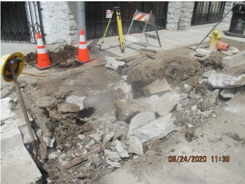
PARK MESA – Excavating for the restoration of Catch Basin #30 on the northeast corner of Crenshaw Blvd and 67th St.
