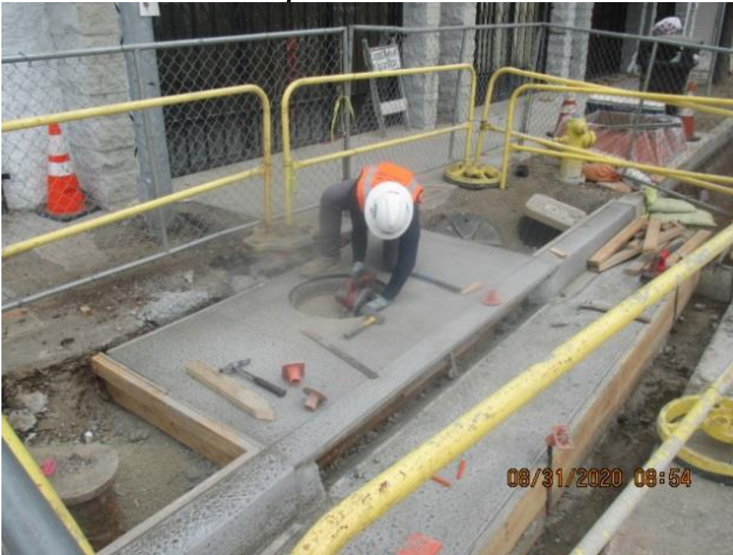
PARK MESA – Sack and patching Catch Basin #30 on the northeast corner of Crenshaw Blvd and 67th St.
