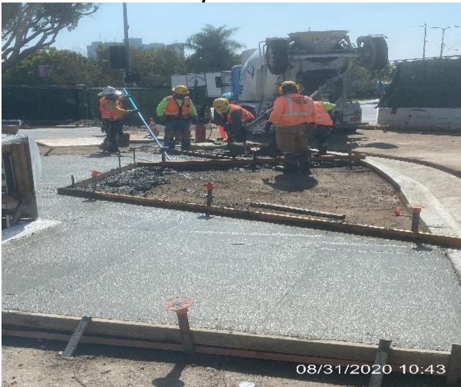
LEIMERT PARK STATION – Built formwork and placed concrete for new ADA ramp (2 of 2) installation on the northeast corner of Crenshaw Blvd and 43rd Pl.
