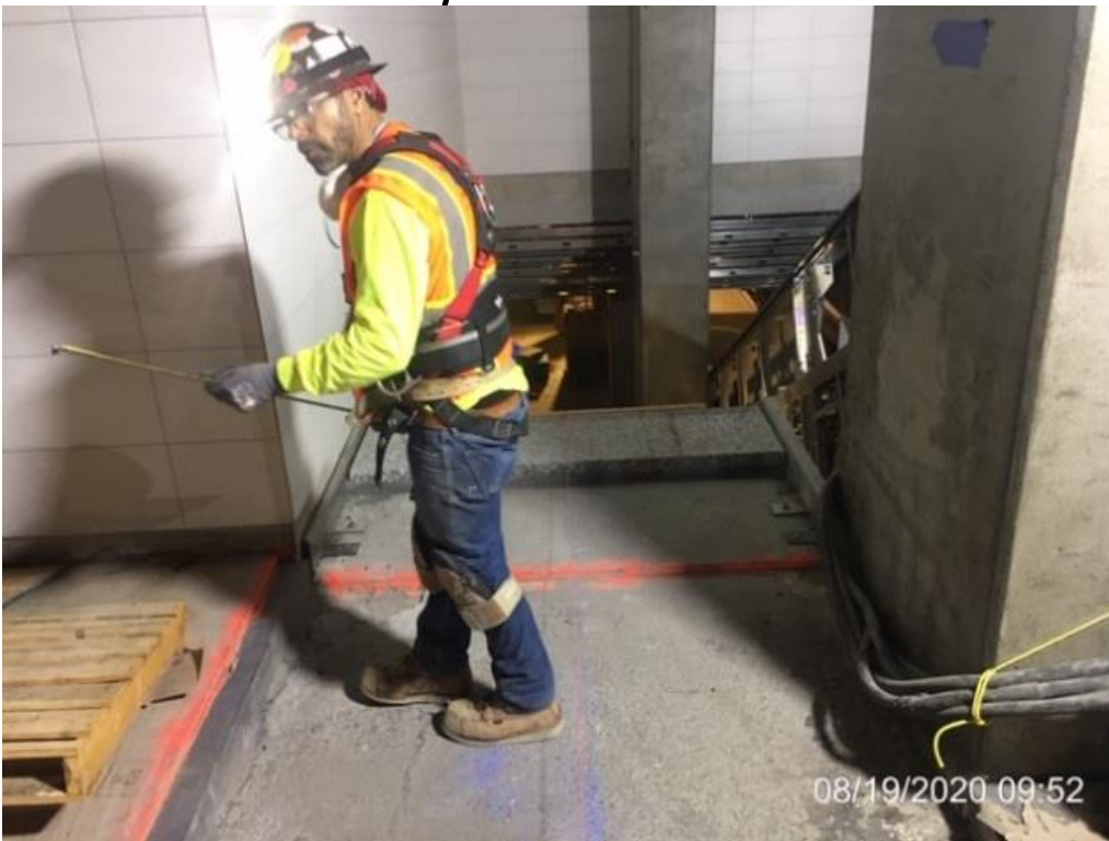
MLK STATION – Preparing and laying out for granite paver installation for the base landings of Staircases 2&3 at the concourse level.
