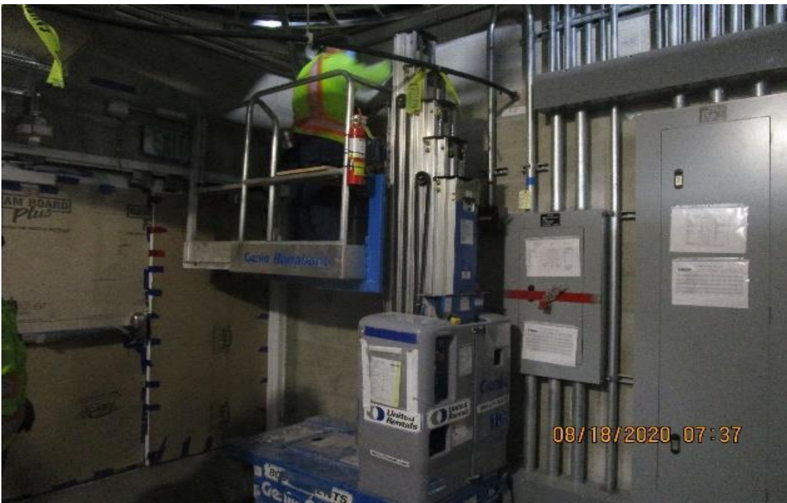
Crenshaw/Vernon – Vernon, Aux power (N) C119, Pipping ¾” GRC from temperature control panel to MCC2/N (control wiring)
