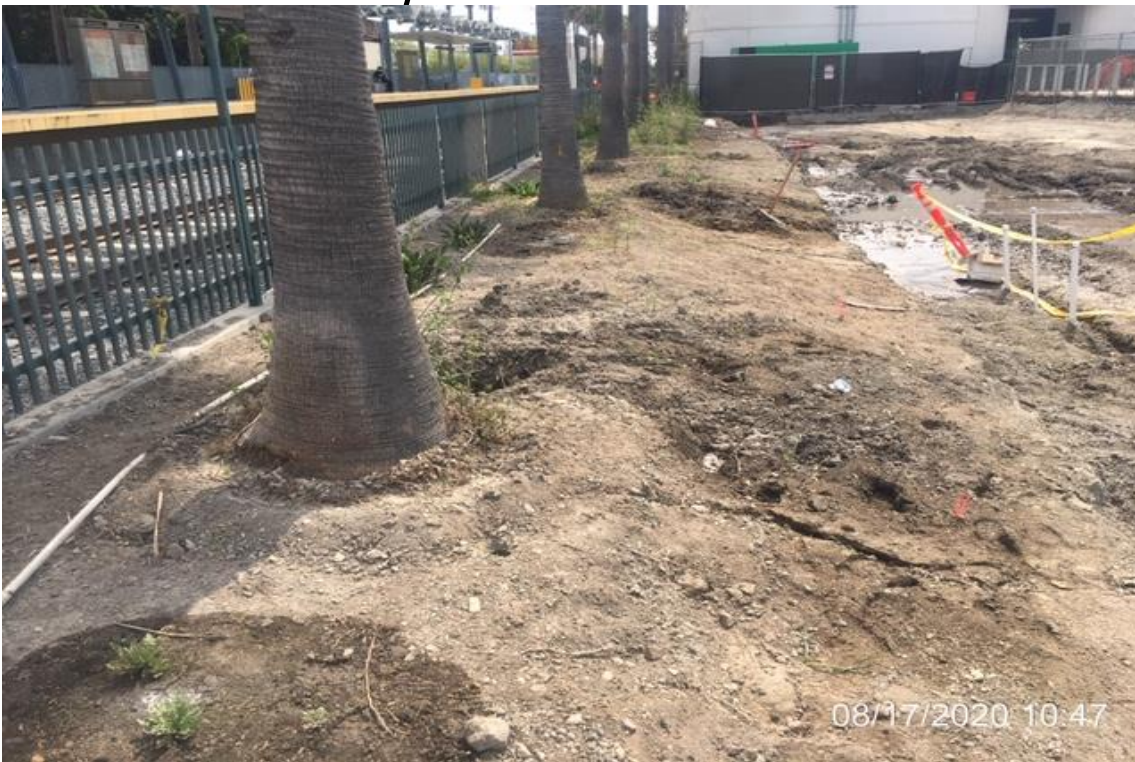
EXPO STATION – active irrigation line continues to soak north yard.
