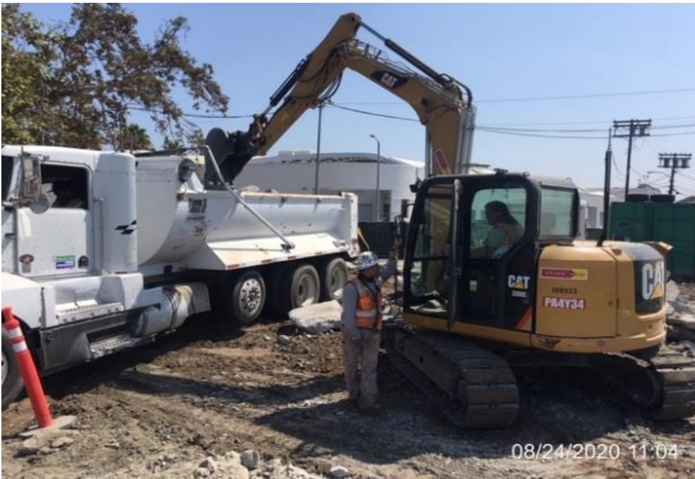
EXPO STATION – Continue demolishing/removing/hauling of existing concrete slab at the northern lot area.
