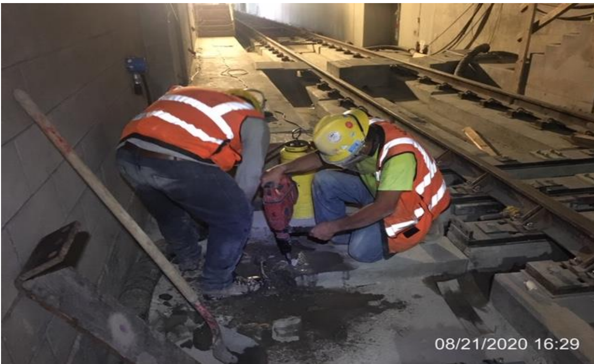
EXPO STATION SITE – WSCC crew demoing plinths that do not meet strength requirement
