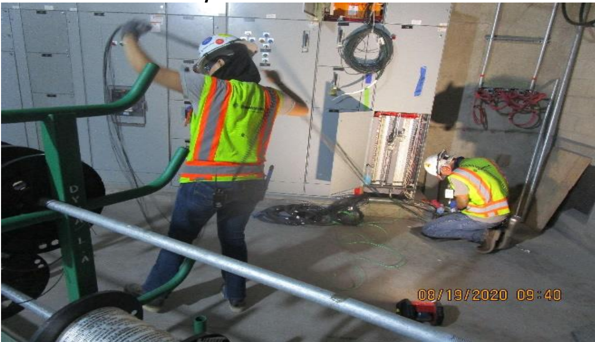
MLK STATION – Aux Power (N) C132, MCC1/N, CIC1/N Pulling damper power & control wiring to LCS for EVF-7-122.
