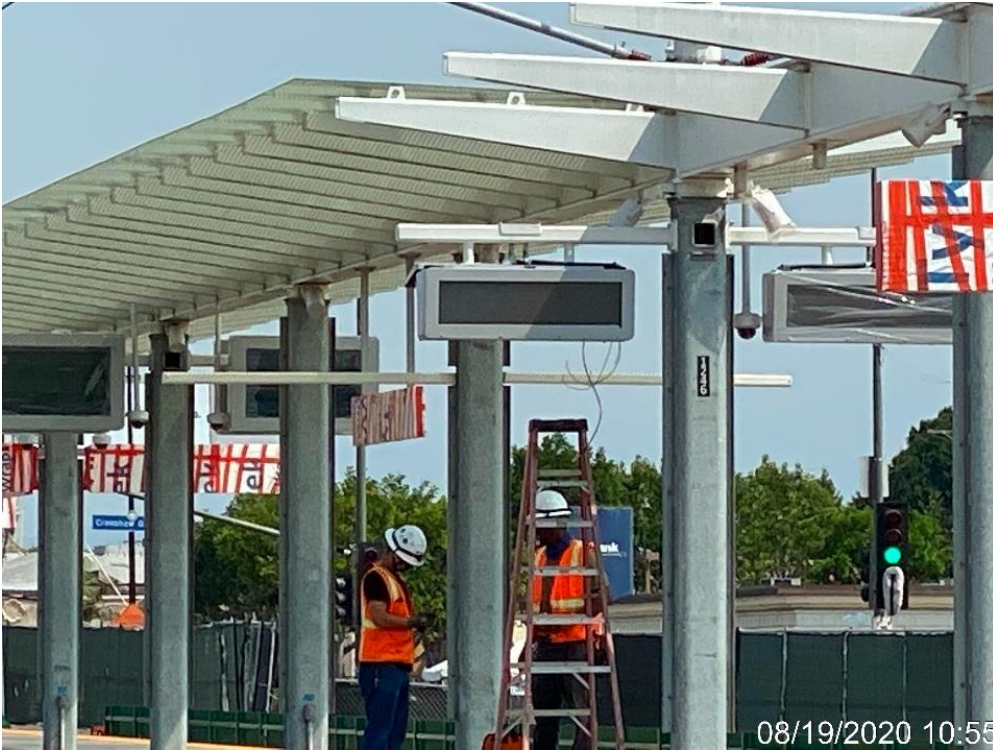
HYDE PARK STATION – Continue installing LCD variable messaging systems at the south end of the platform level.
