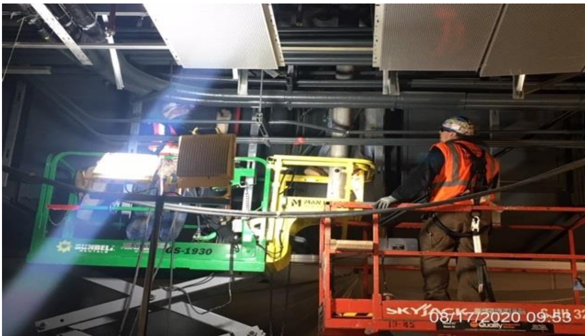
MLK STATION – WSCC ironworkers welding down stands on SB side of platform.
