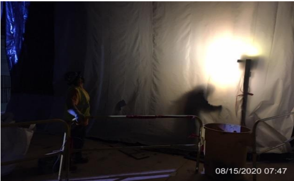
EXPO STATION SITE – McMahon sandblasting HSS fascia of elevator #3 and #4 at platform level.
