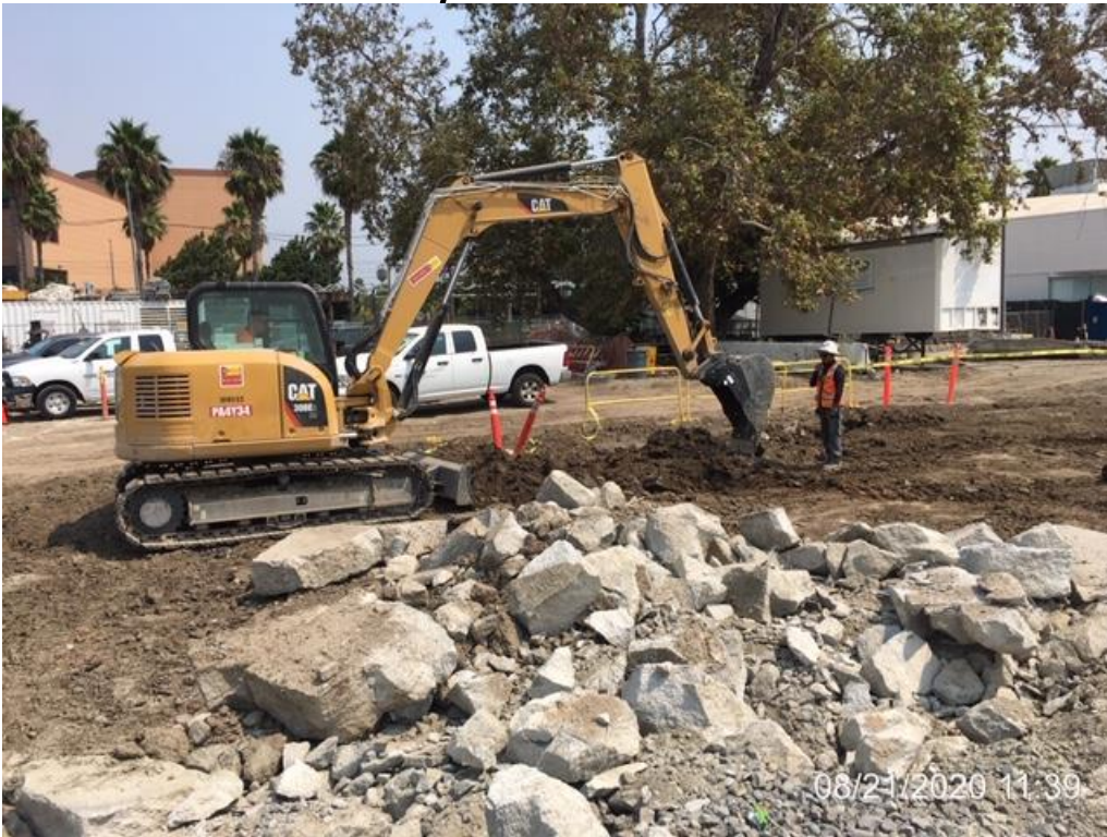
EXPO STATION – Continue demolishing/removing/hauling of existing concrete slab at the northern lot area.
