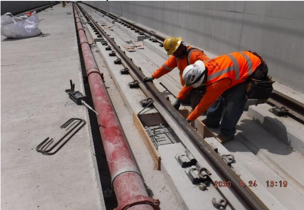
UG3 – STA 277+50 TK#3/SB looking south – NCR-A-111.B Case #4 UG3 new dowel epoxy (Victoria)
