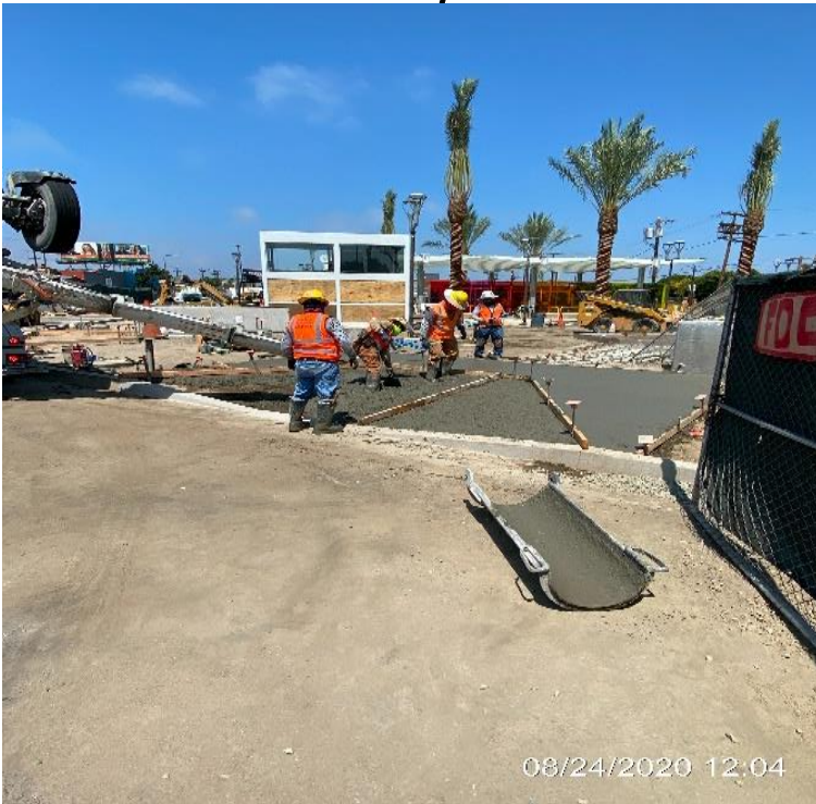
LEIMERT PARK STATION – Built formwork and placed concrete for new ADA ramp (1 of 2) installation on the northeast corner of Crenshaw Blvd and 43rd Pl.
