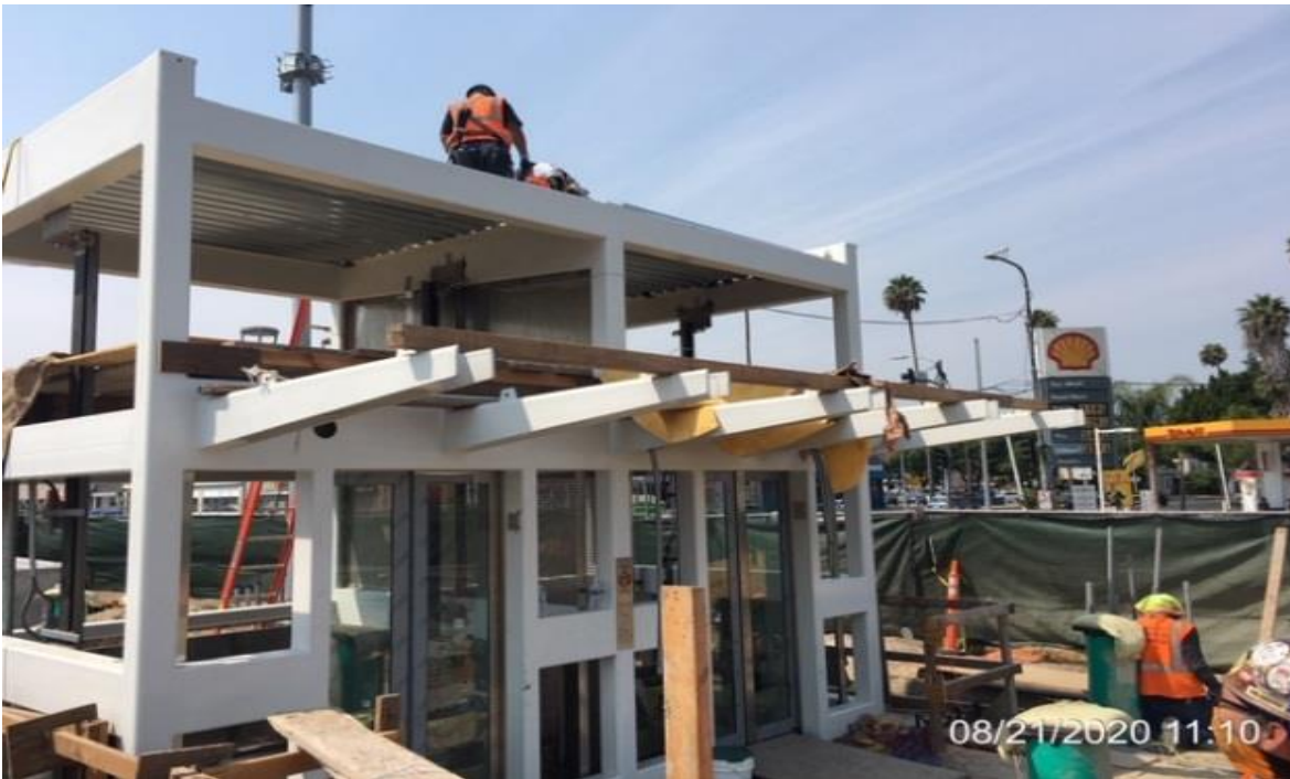
EXPO STATION SITE – Ironworkers installing metal roof decking on elevator structure #1 and #2.
