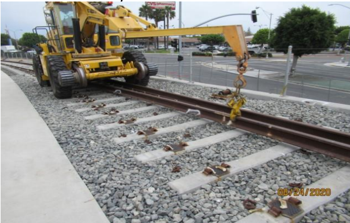
La Brea – HCC using speed swing & rail dogs to remove rails on NB track at La Brea wall 202 between STA 203+ 50 & 207+50 (looking northeast) Rework
