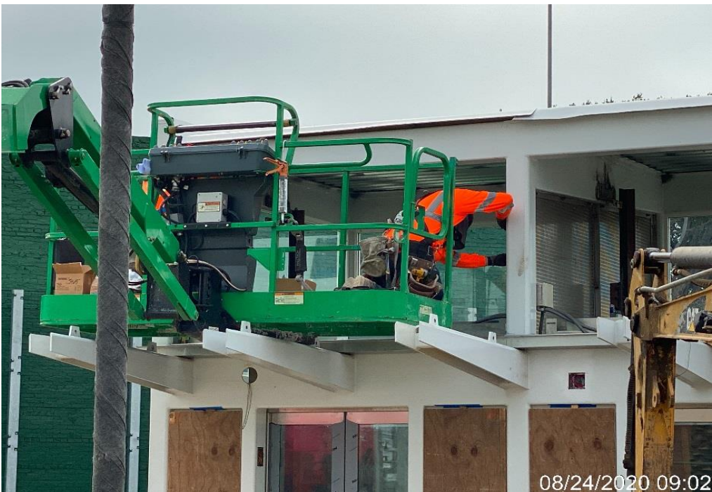
LEIMERT PARK STATION – Installing ventilation louvers to Elevators 1&2 at the plaza level.
