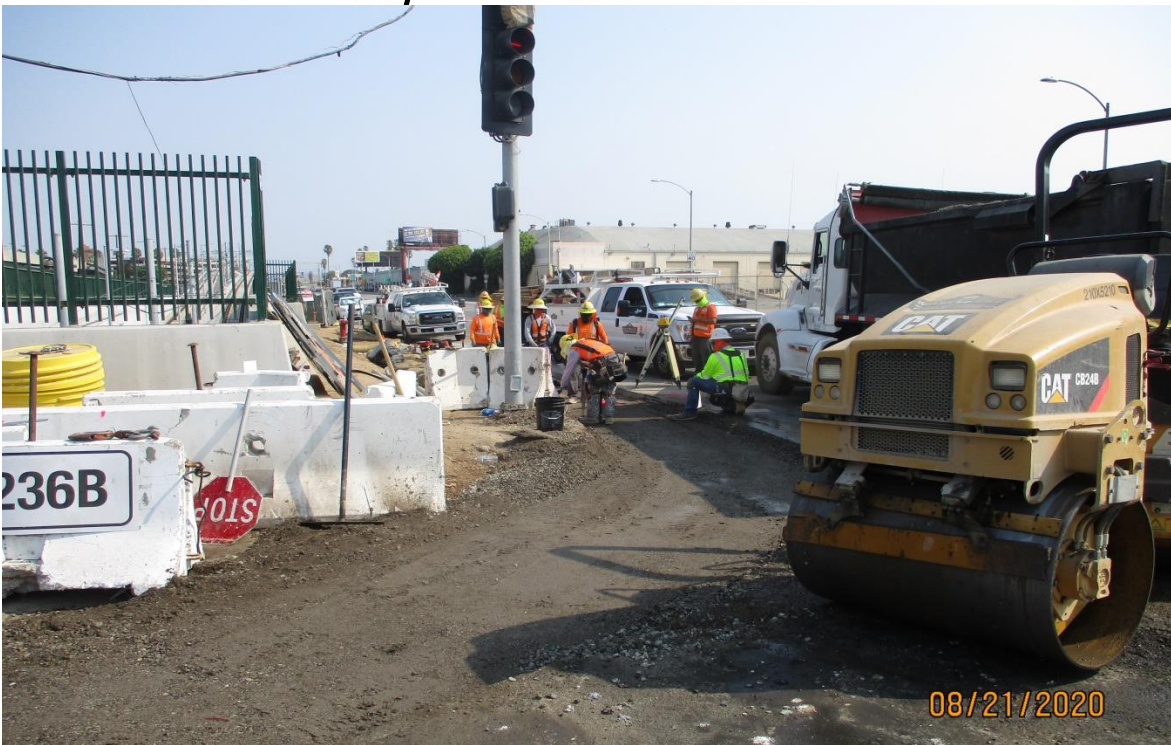
AVIATION/CENTURY- Grading, compaction and setting forms for the curb and gutter on Aviation near 104th street.
