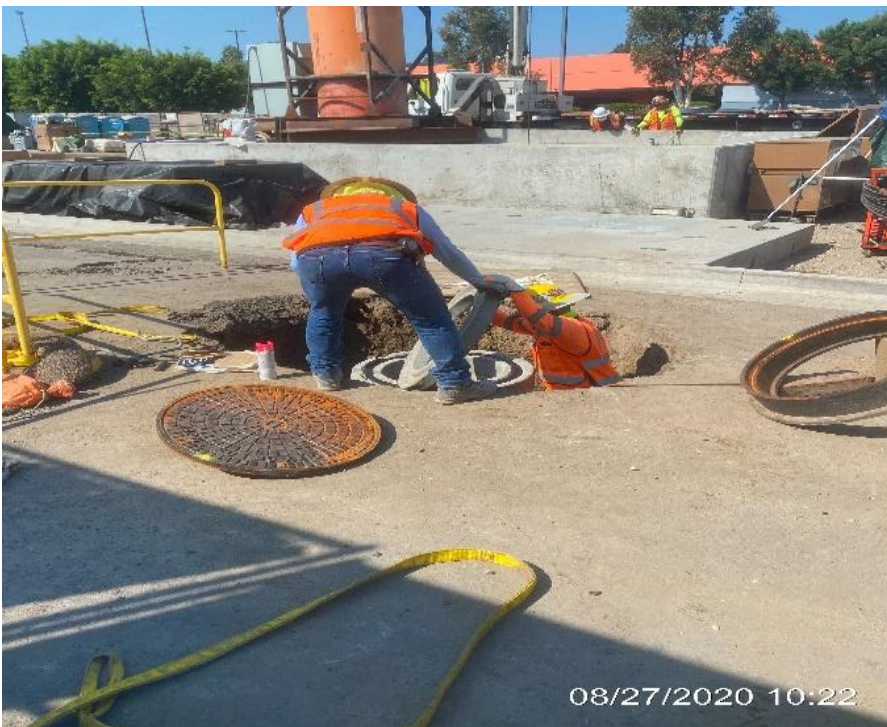
MLK STATION – Installing lid and risers inside Manhole #18 at the plaza level.
