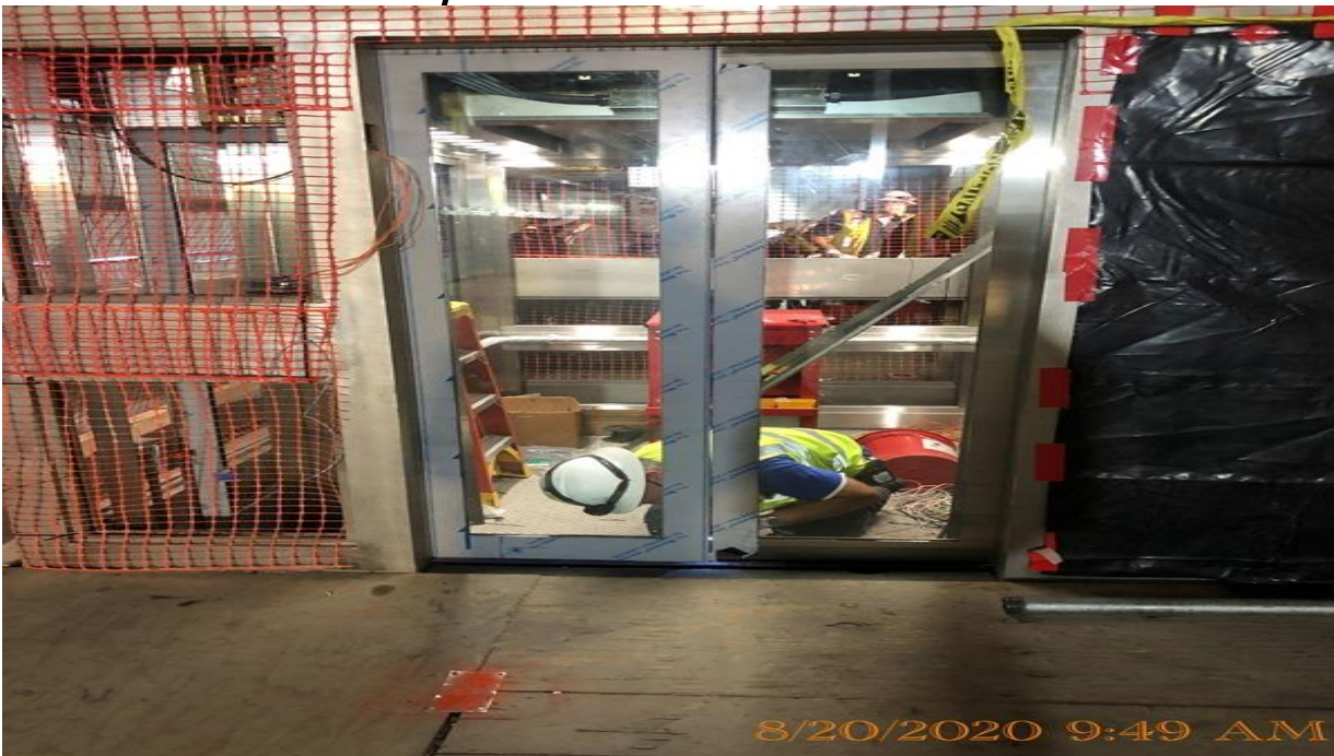
EXPO STATION – Continue final wiring and adjustments for all 4 Elevators at the concourse level.
