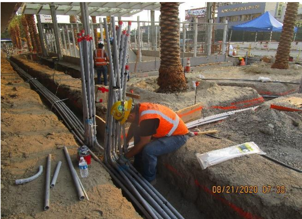
MLK STATION – Continue installing conduit for landscape lighting throughout the plaza level.
