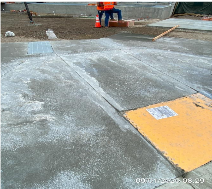
LEIMERT PARK STATION – Saw cut ADA ramp entrance (2 of 2) into the station plaza on the northeast corner of Crenshaw Blvd and 43rd Pl.
