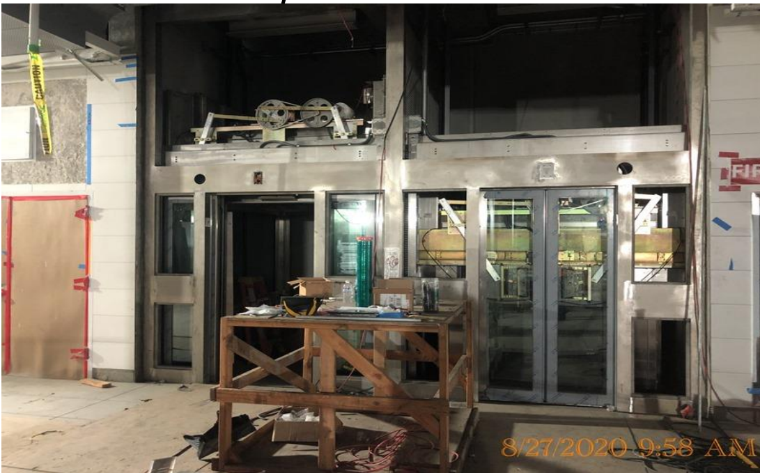
EXPO STATION – Continue final wiring and adjustments for Elevators 1&2 at the concourse level.
