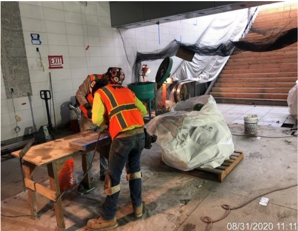
MLK STATION – Continue installing granite pavers to the bottom landing of Staircase 1
