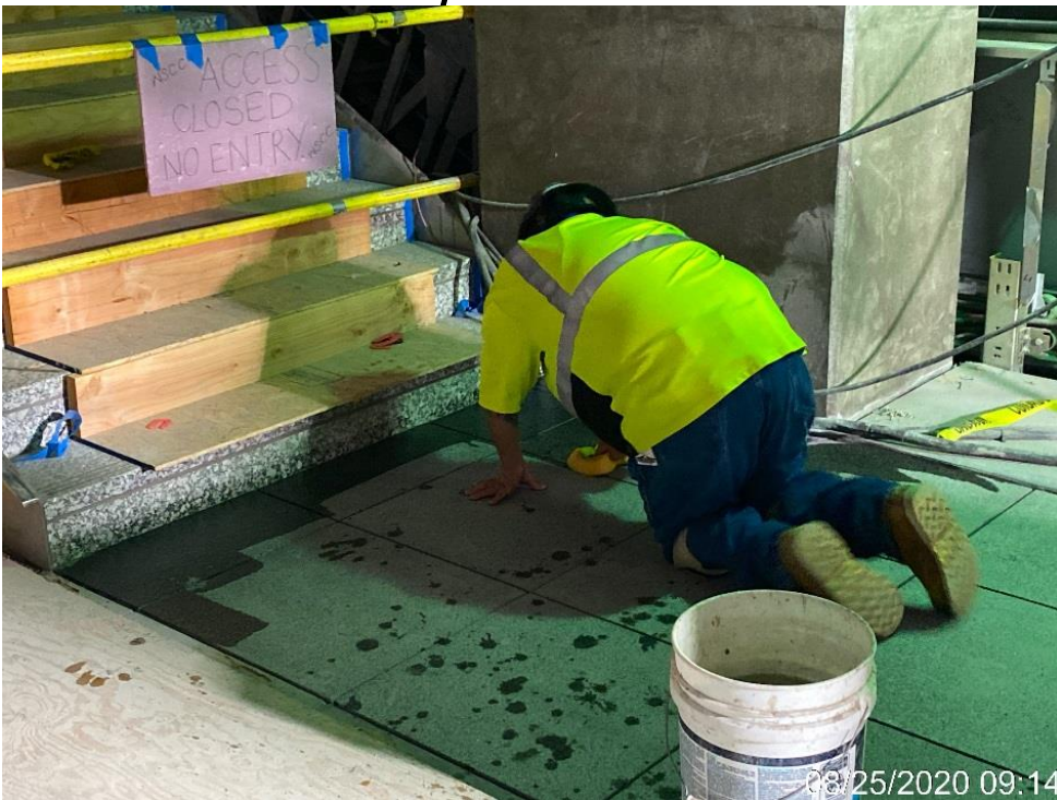
LEIMERT PARK STATION – Grouting granite pavers on the base landing of Staircase #4 at the platform level.
