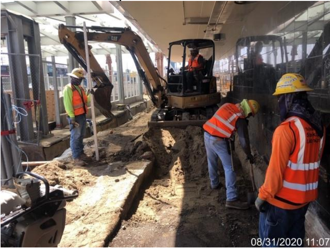
MLK STATION – Backfilling/compacting walkway adjacent to Mall building at the plaza level.
