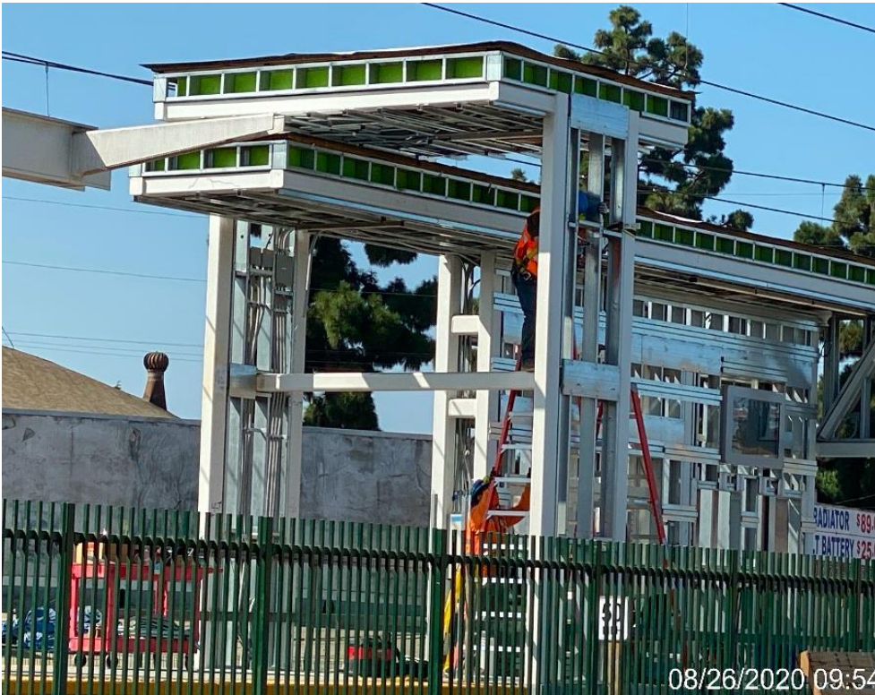
HYDE PARK STATION SITE – Continue installing roofing to the canopy on the south end of the platform level.
