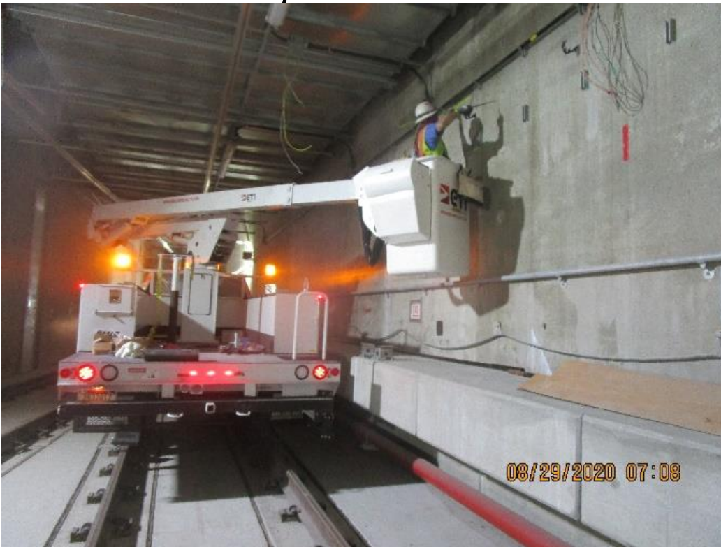
EXPO STATION – Continue installing supports and fixtures for the crossover lighting at the invert level.
