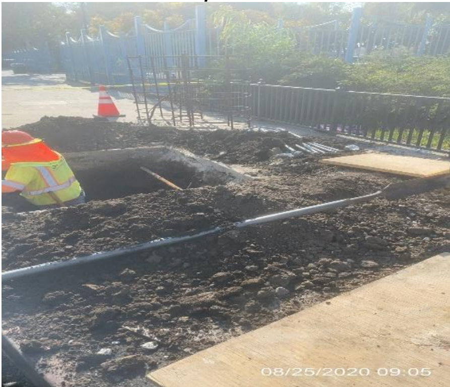
LEIMERT PARK STATION – Preparing to form street light pole foundation on the southeast corner of Crenshaw Blvd and 43rd Pl.
