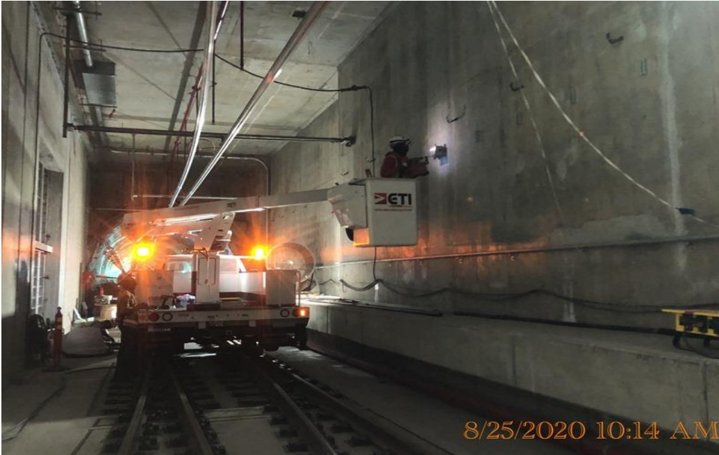
EXPO STATION – Continue installing supports and fixtures for the crossover lighting at the invert level.
