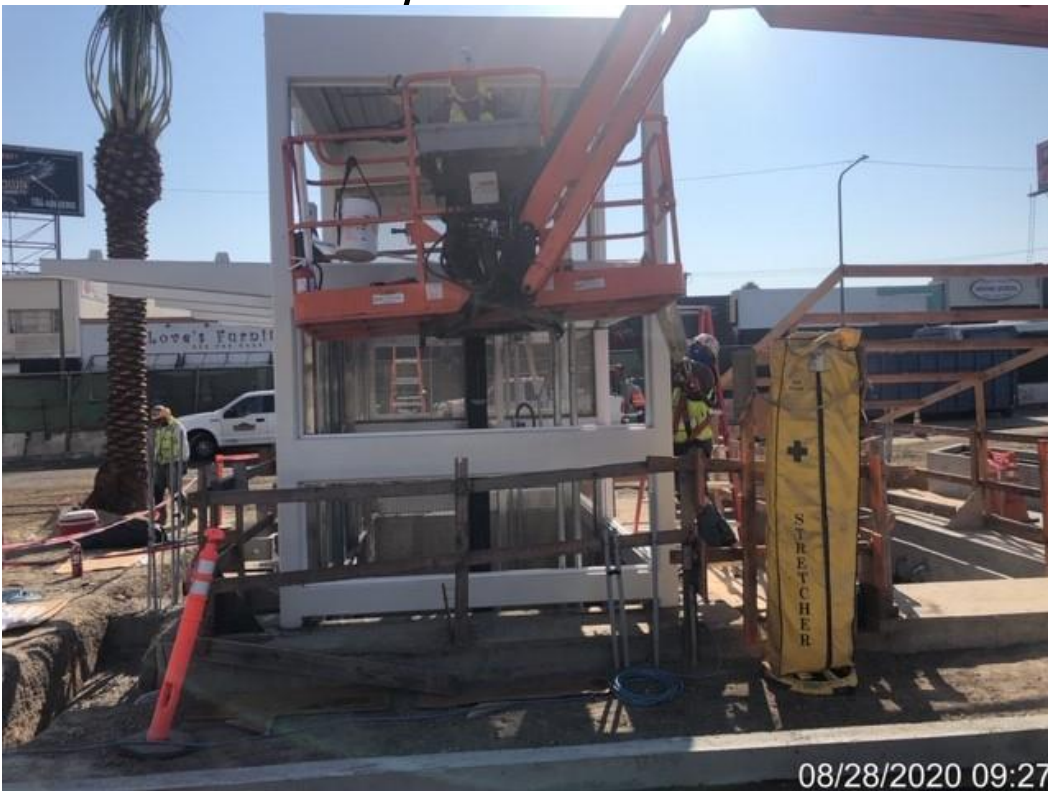
MLK STATION – Continue installing glass hardware in preparation for glass panel installation to Elevators 1&2 at the plaza level.
