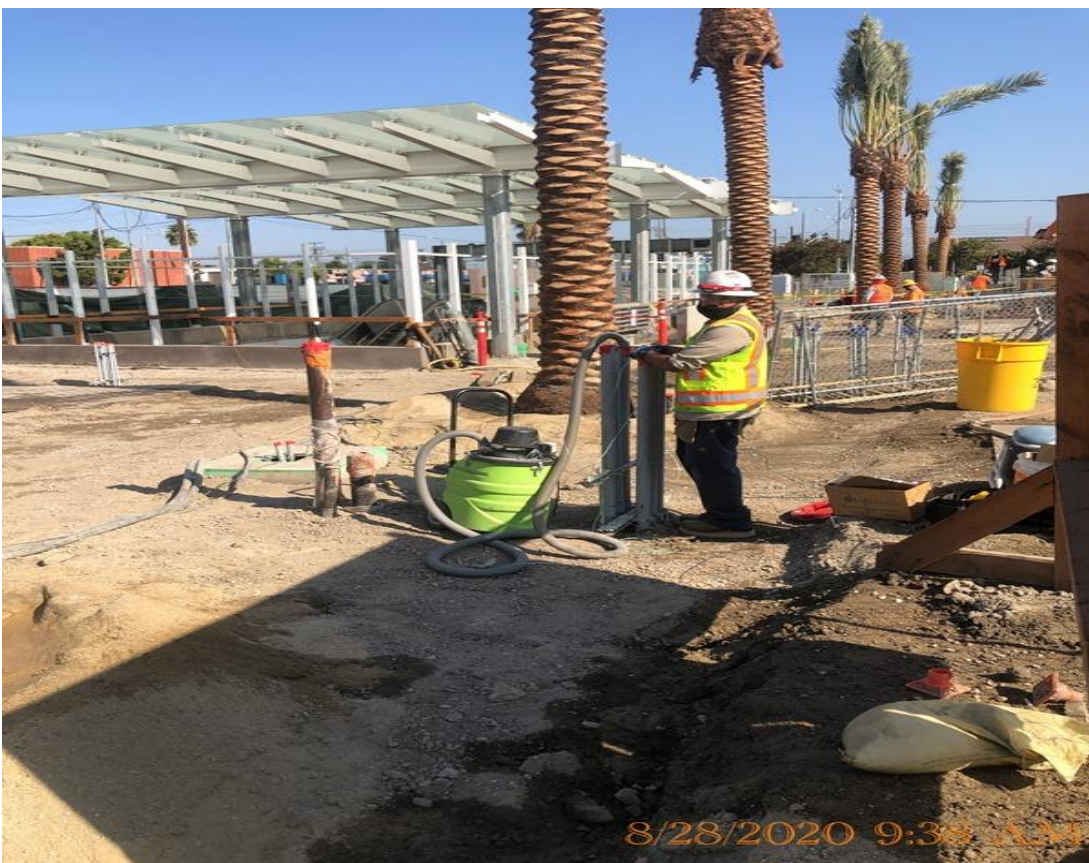
EXPO STATION – Continue installing conduit for landscape lighting at the plaza level.
