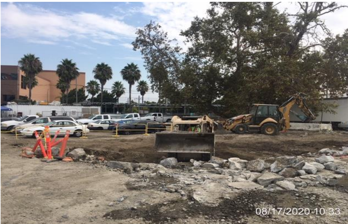
EXPO STATION - WSCC crew removing concrete slab from east side of yard.
