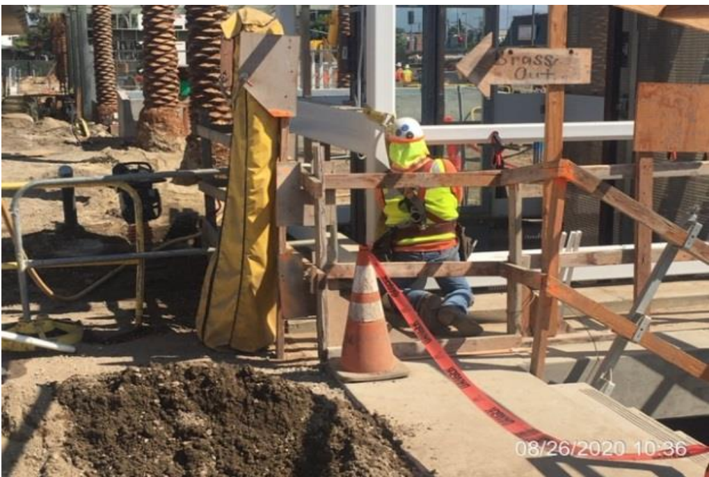
MLK STATION – Installing glass hardware in preparation for glass panel installation to Elevators 1&2 at the plaza level.
