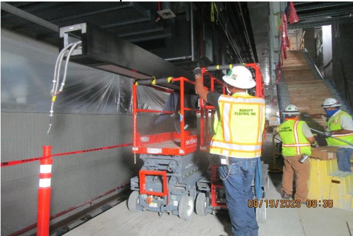
Crenshaw/Vernon – Vernon Platform, SB GL's 8-9/C, begin hanging & anchoring edge lighting to support post SB track #3
