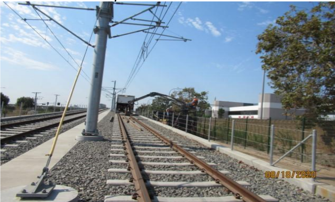
Guideway- HCC on SB track staging switch points for T/O's that will be replaced at GL Wye (looking south) Rework
