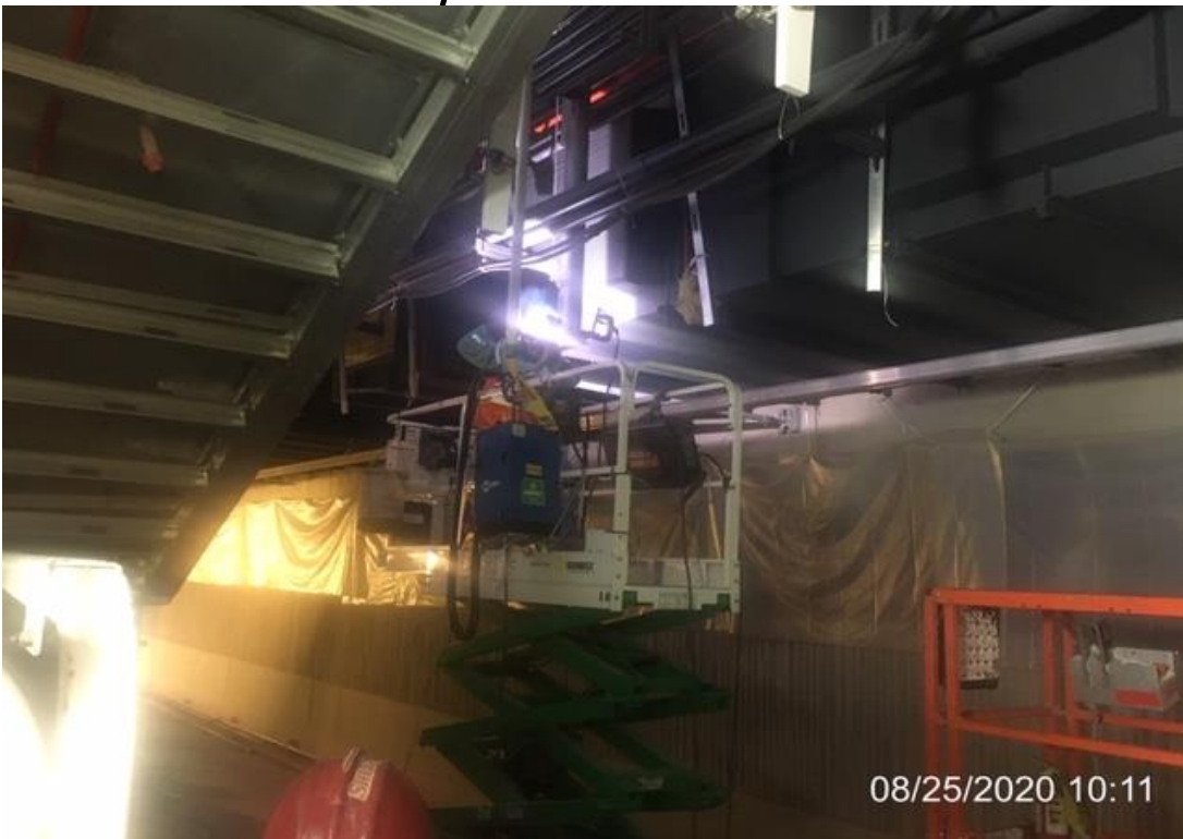
MLK STATION – Continue welding edge plates to the down stand support poles on both the north and southbound sides of the platform level.
