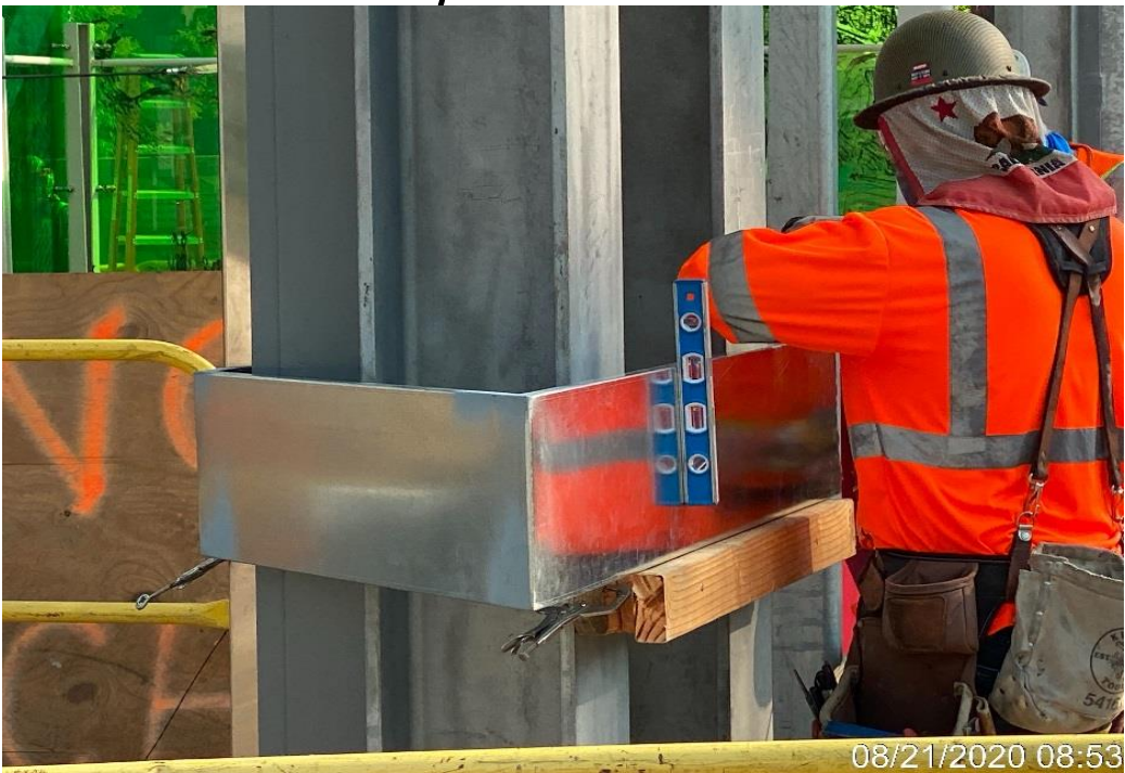
LEIMERT PARK STATION – Building column cover mock-up at the main entrance canopy structure at the plaza level.
