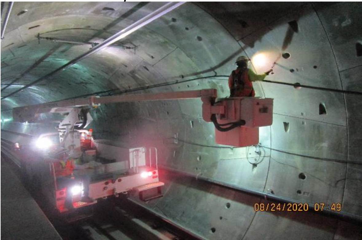
Crenshaw/Vernon – Bored Tunnel, SB, Vernon to MLK, North of CP5, West side of tunnel liner resume pulling 1-1/4” Radiax cable
