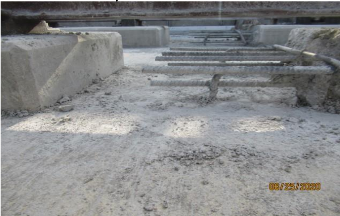
AVIATION/CENTURY- Excavating for the traffic signal conduit on Aviation north of Century.
