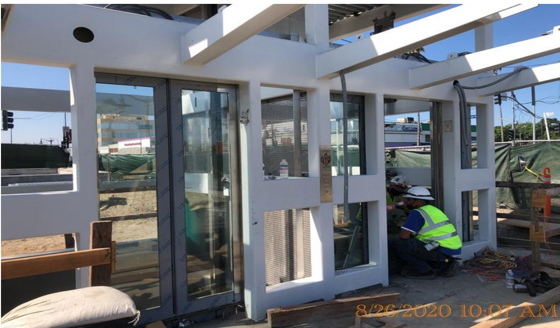
EXPO STATION - Setting supports for floor drainage at the main entrance portal of the plaza level.
