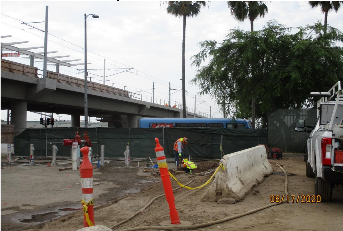
AVIATION/CENTURY- Installing the copper irrigation pipe at the Aviation Station plaza area.
