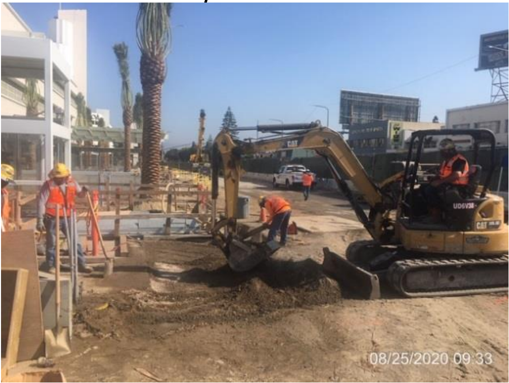
MLK STATION – Backfilling concrete landscape conduit duct banks trenches on the east side of the plaza level.
