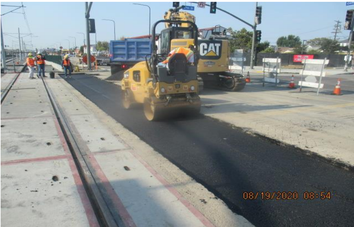
PARK MESA – Placing asphalt concrete roadway cap on the intersection of southbound Crenshaw Blvd and 57th St.
