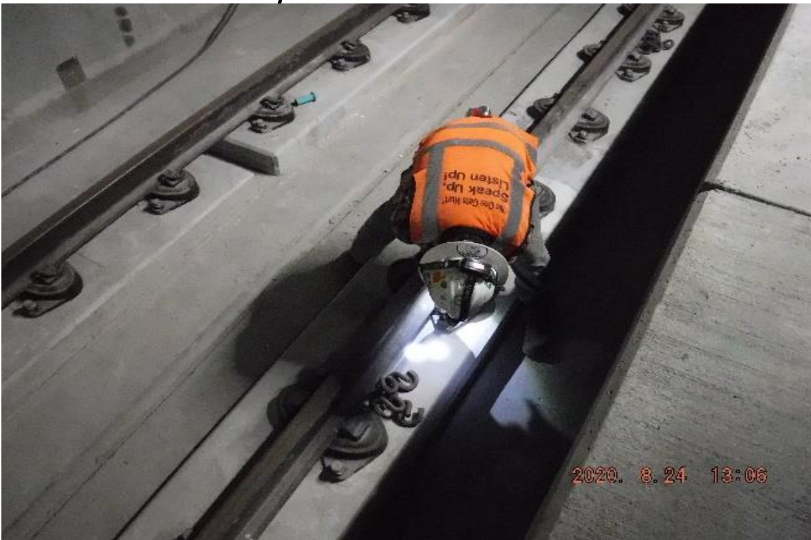
UG3 – STA 302+20 TK#3/SB looking north – NCR-A-111.B Case #4 UG3 (re-set DF's anchor bolts)
