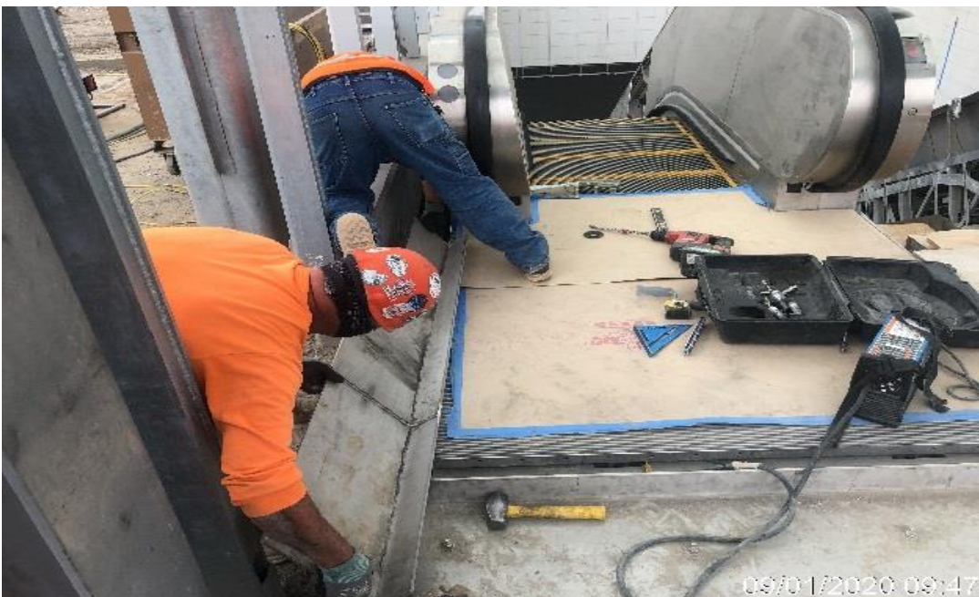
EXPO STATION – Installing bent plates to Escalators 1&2 at the main entrance portal of the plaza
