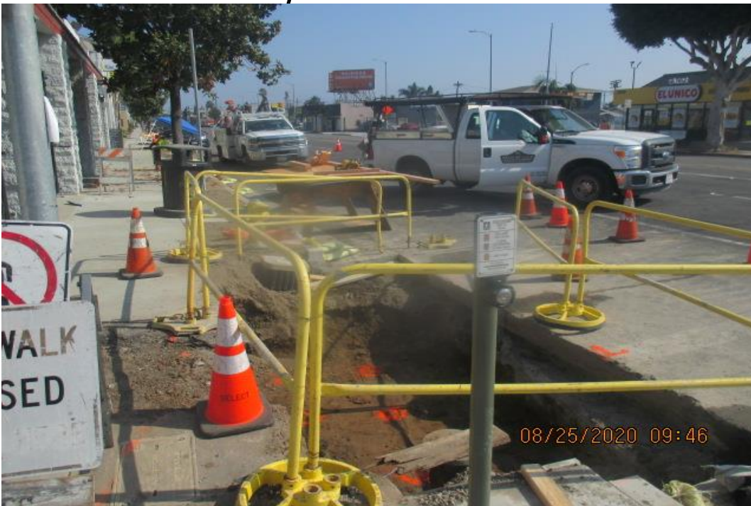
PARK MESA – Building stem wall forms for Catch Basin #30 on the northeast corner of Crenshaw Blvd and 67th St.
