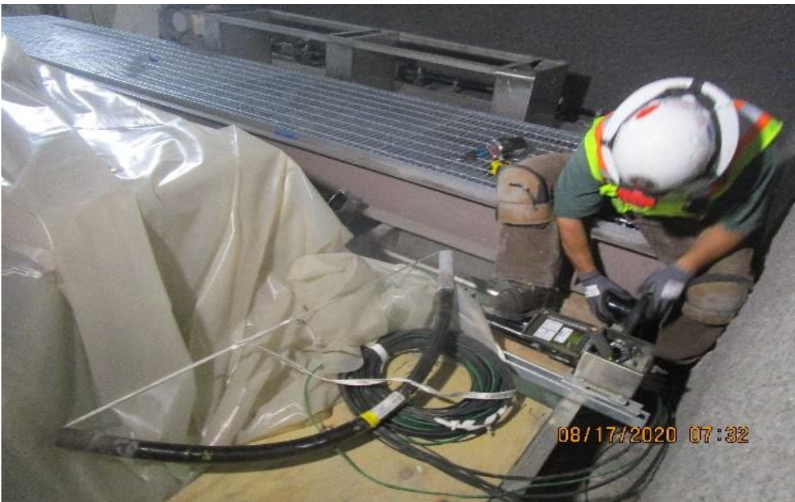
Crenshaw/Vernon – Vernon, Emergency fan room (S) C102, begin rework OTED's 6-301 & 101 replace seal tight with 1" FRP.
