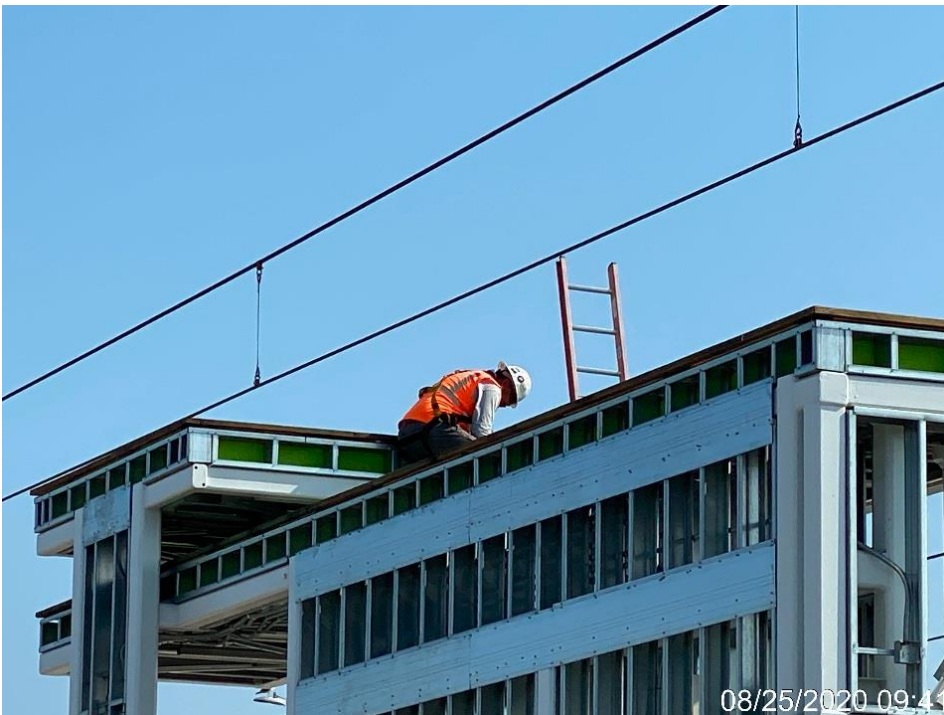
HYDE PARK STATION – Installing roofing to the canopy on the south end of the platform level.
