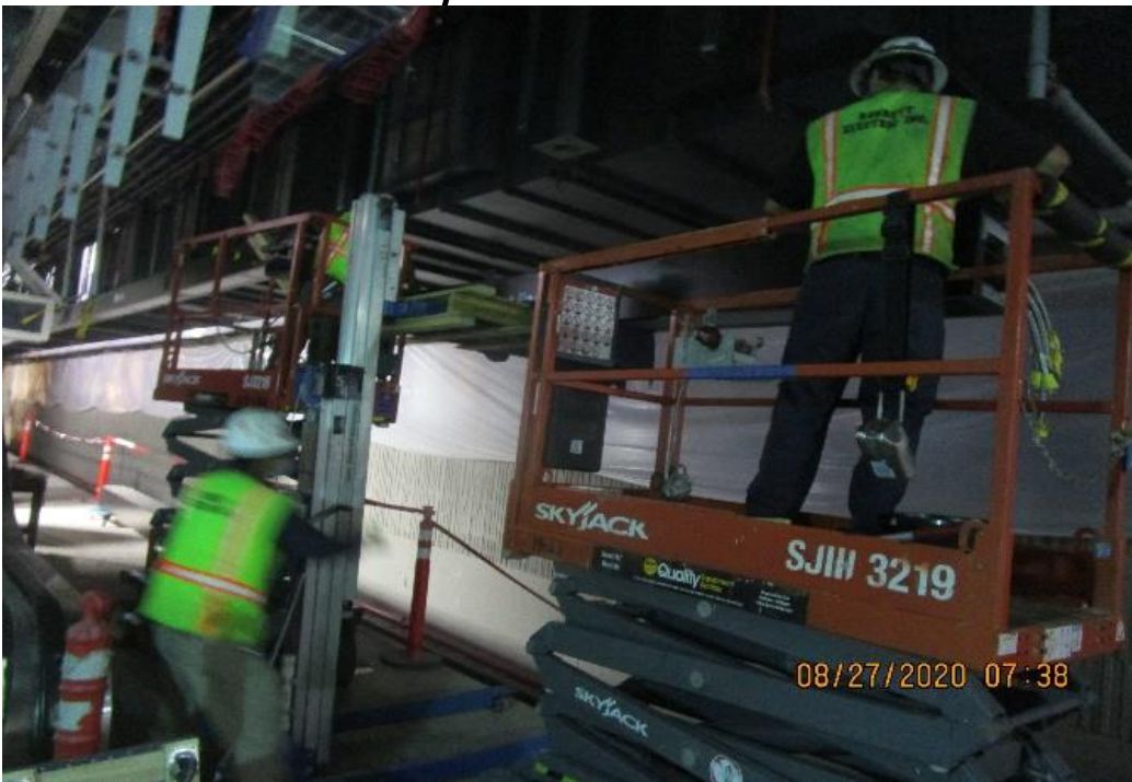
LEIMERT PARK STATION – Continue installing edge lights to the down stand support poles on the northbound side of the platform level.
