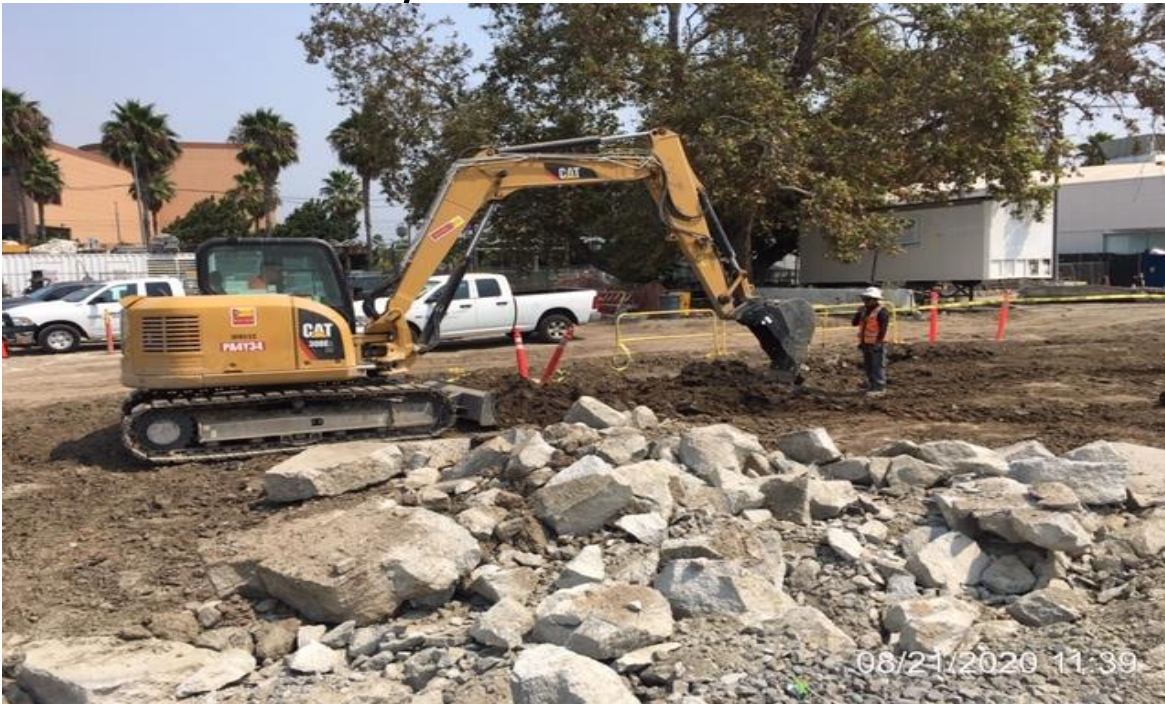
EXPO STATION SITE – WSCC crew demoing existing concrete slab and foundation for removal.
