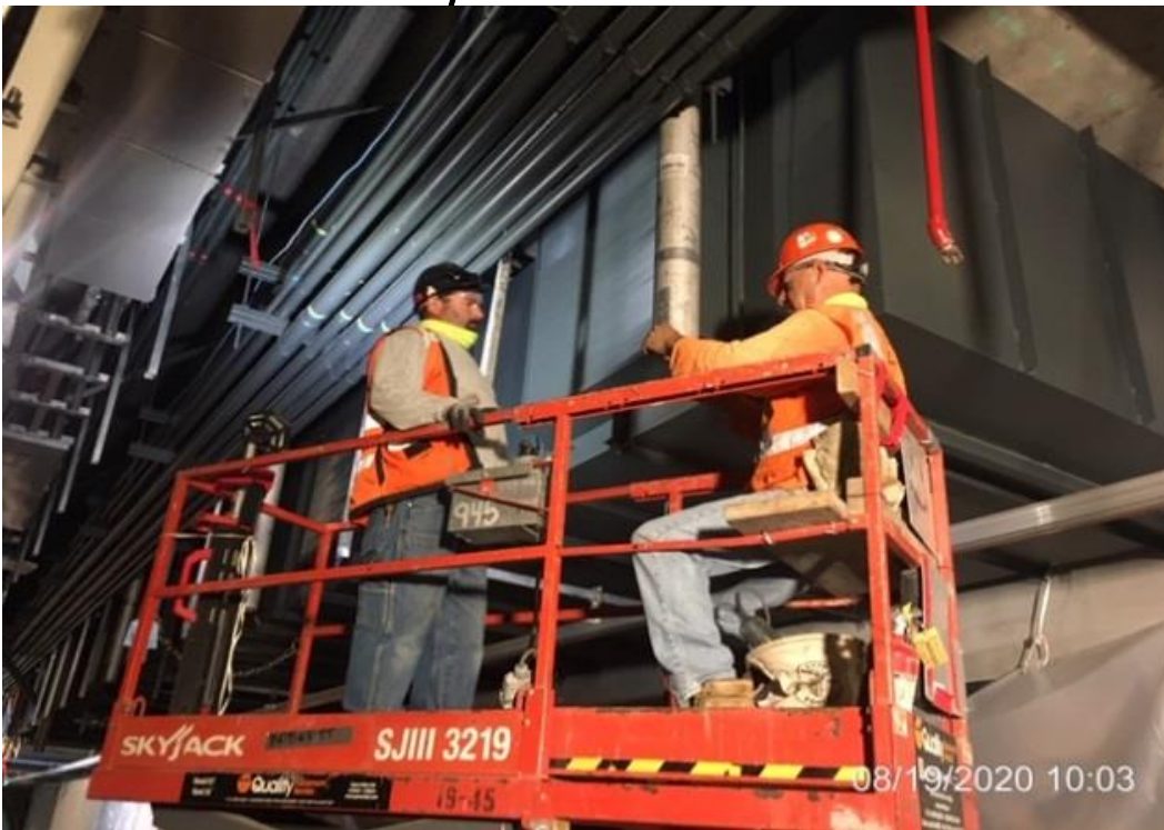
MLK STATION – Continue welding down stand support poles and sleeve joints on both the north and southbound sides of the platform level.
