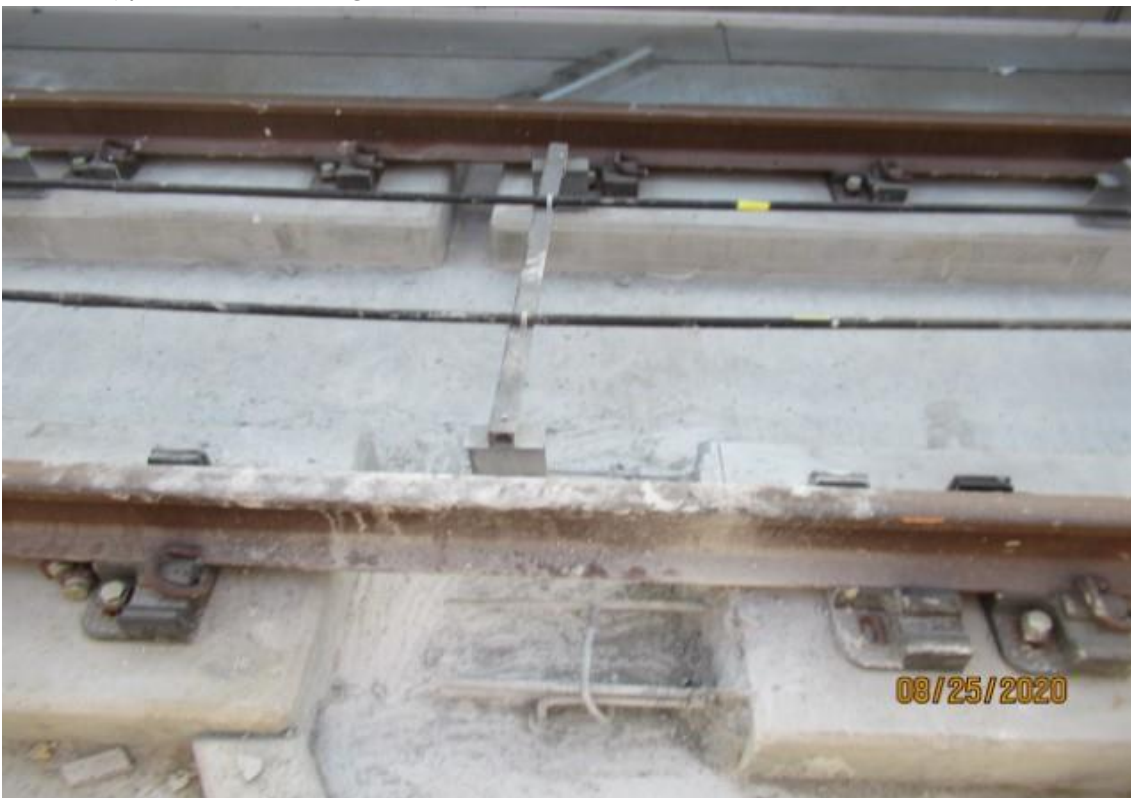
AVIATION/CENTURY- SB track left plinth where WSCC previously demoed end of plinth for rebar dowel install at Century/Aviation station platform
