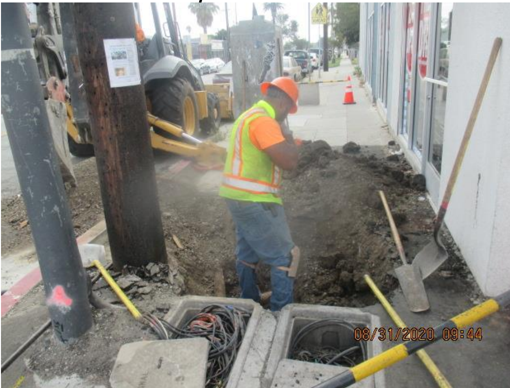
PARK MESA – Excavating for pull box installation for new street and signal light poles the southeast corner of Crenshaw Blvd and Hyde Park Blvd.
