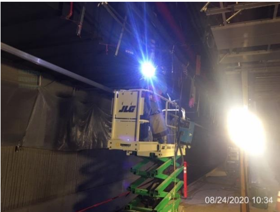
MLK STATION – Continue welding edge plates to the down stand support poles on both the north and southbound sides of the platform level.
