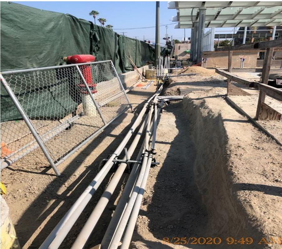
EXPO STATION – Continue installing conduit for landscape lighting on the west side trenches of the plaza level.
