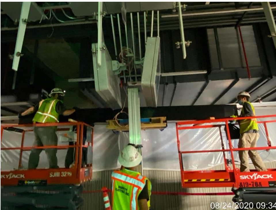
LEIMERT PARK STATION – Continue installing edge lights to the down stand support poles on the northbound side of the platform level.
