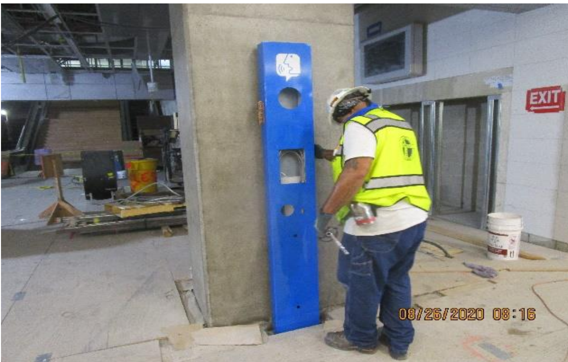
Crenshaw/Vernon – Vernon Concourse, Paid Area C146, begin anchoring ETEL, PTEL podium enclosures & at platform level
