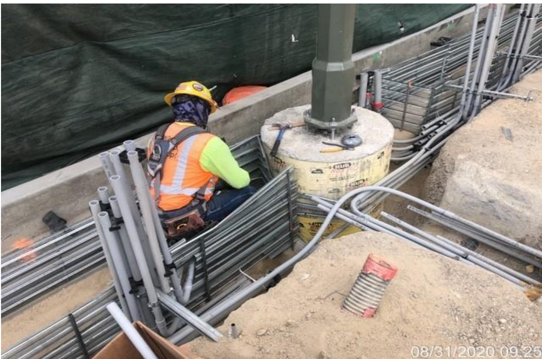
EXPO STATION – Setting formwork in preparation for concrete encasement for the west side conduit landscape trenches of the plaza level.
