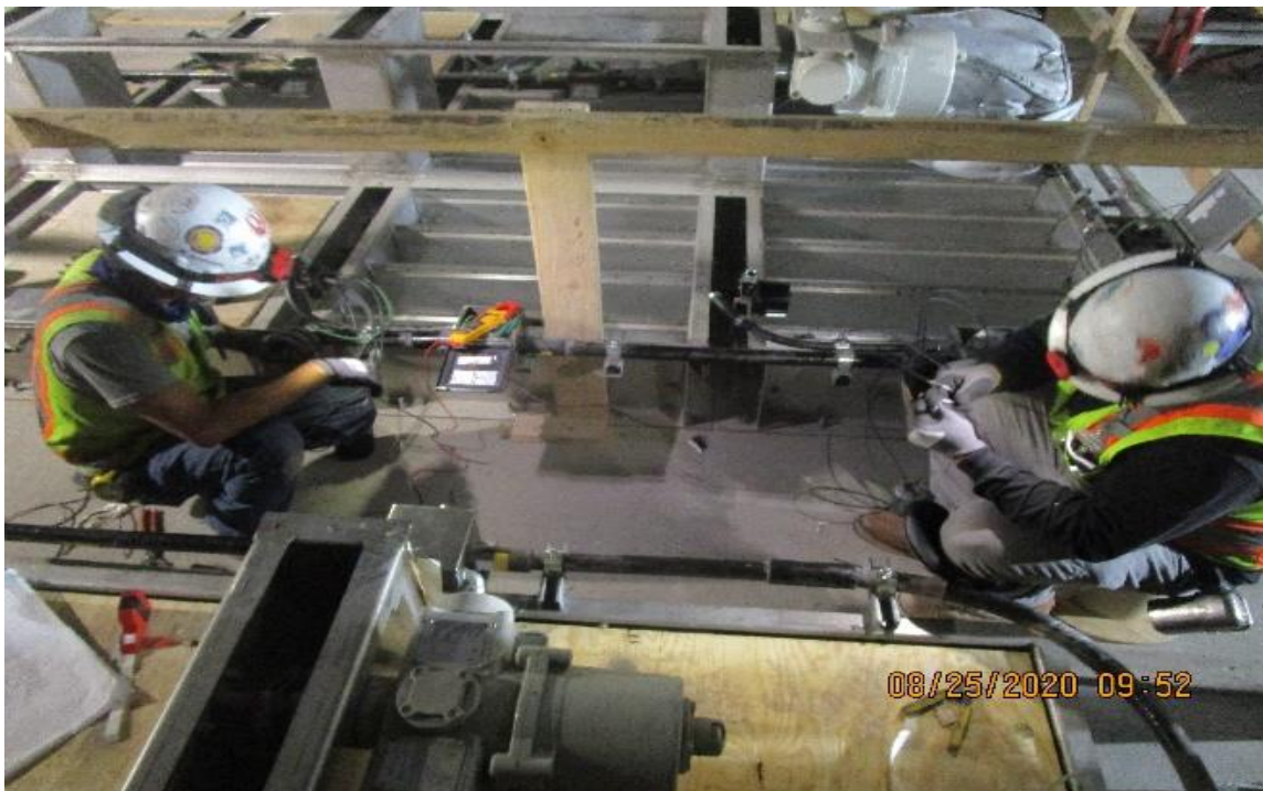
MLK STATION – EM Fan (s) C102, Pulling jumpers (#14`S RHW-2 & #10 Gnd) TD-7-321 limit switches & continuity testing.
