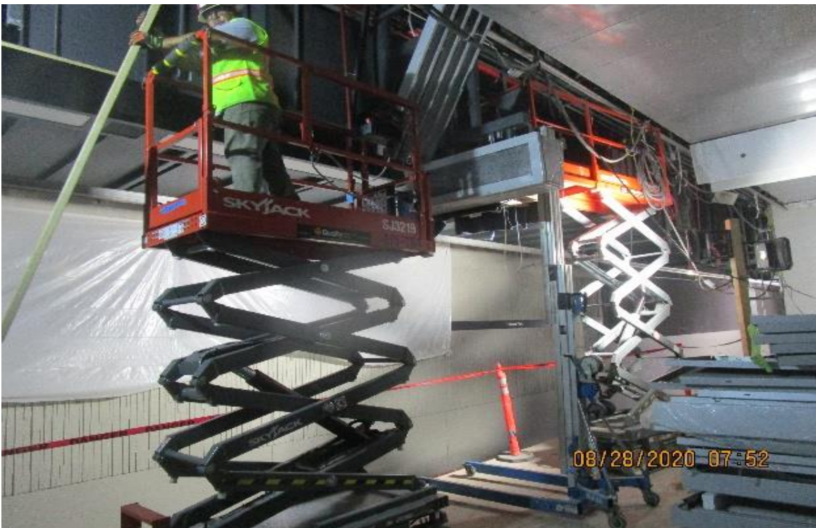
Crenshaw/Vernon – Vernon Platform, SB GL's 13-15/A.5. Continued plumbing, squaring & leveling Edge lighting fixtures.
