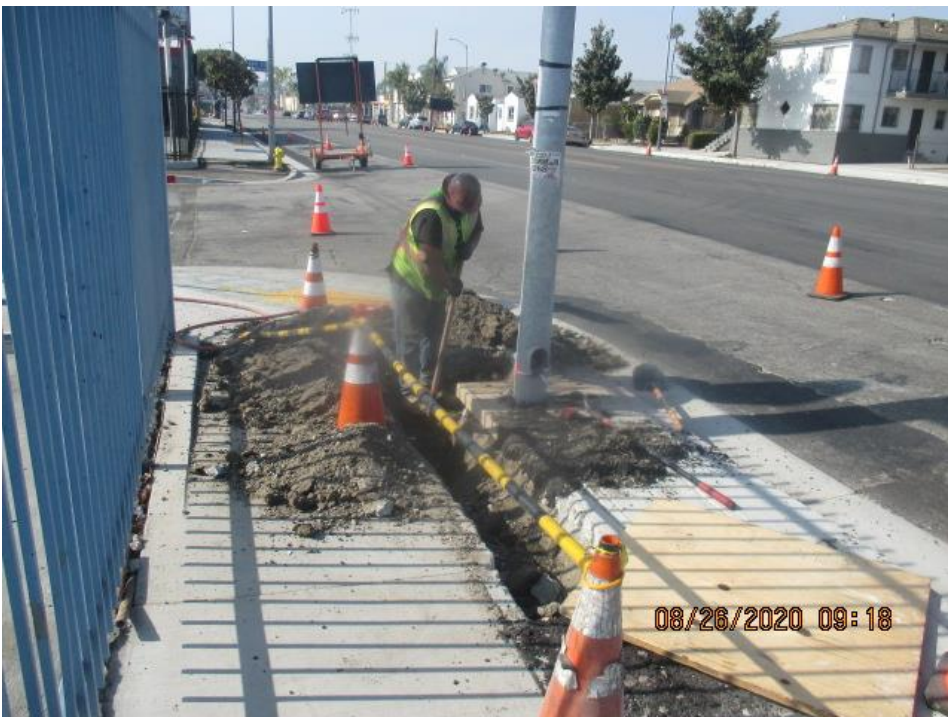
PARK MESA – Excavating for pull box installation for new street light pole on the northeast corner of Crenshaw Blvd and 66th St.
