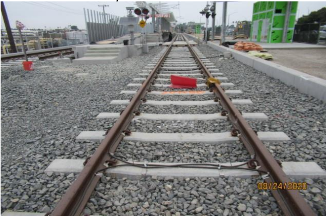
La Brea – NB track La Brea STA 207+25 electrical wiring still in place, with track scheduled for removal at this location (looking north)
