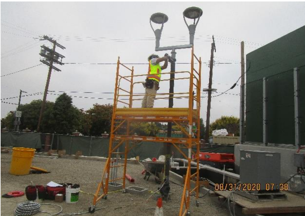
LEIMERT PARK STATION – Installing CCTV cameras to the pedestrian light poles at the plaza level.
