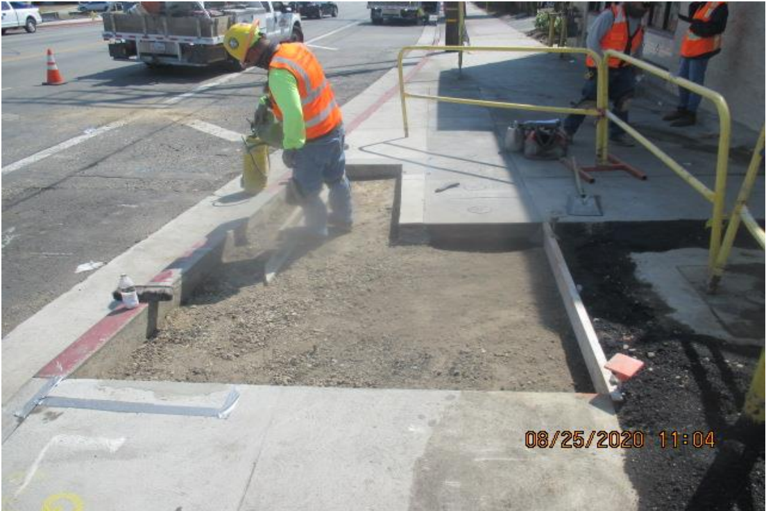
PARK MESA – Demolishing sidewalk panel for restoration on eastbound Slauson Blvd and Crenshaw Blvd.
