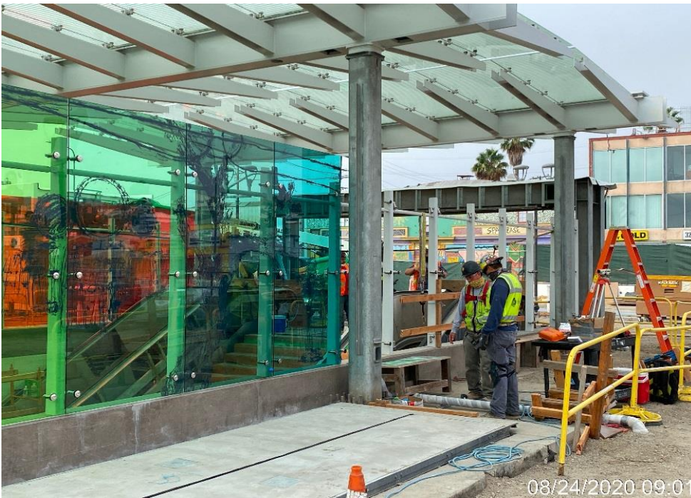
LEIMERT PARK STATION – Continue installing art glass panels around the main entrance canopy structure at the plaza level.
