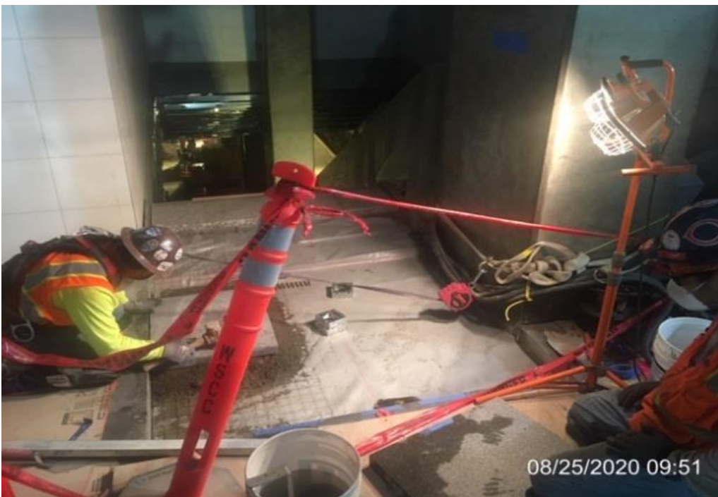
MLK STATION – Installing granite pavers to the base landings of Staircases #2 at the concourse level.
