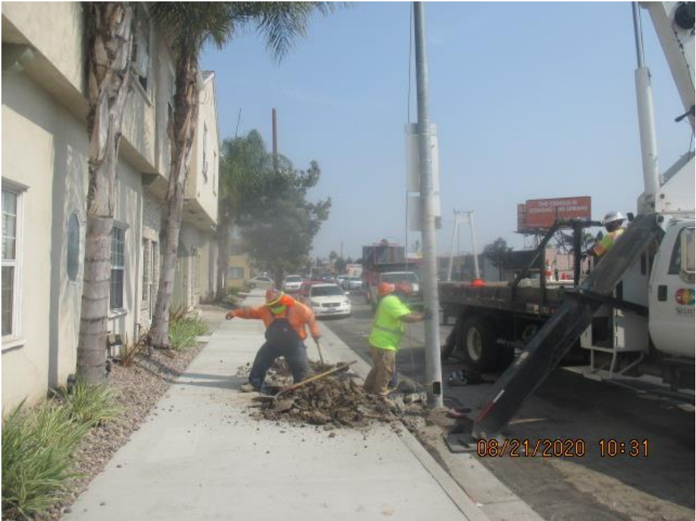
Park Mesa – Excavating for new street light pole foundation on southbound Crenshaw Blvd and 67th St.
