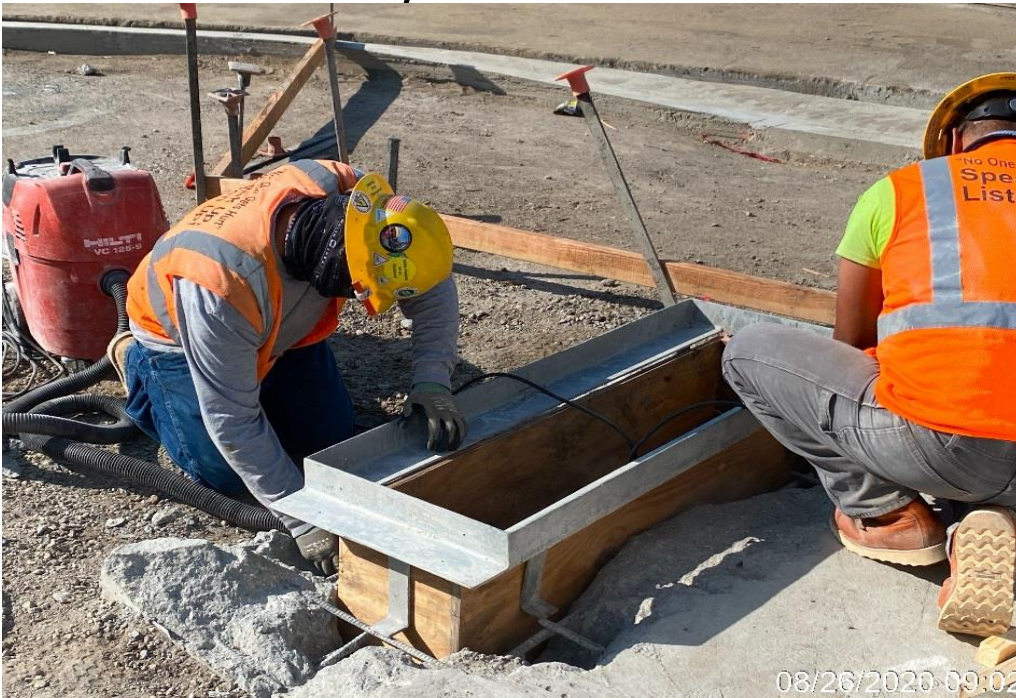
LEIMERT PARK STATION – Building formwork for the Methane Vent Installing at the plaza level.
