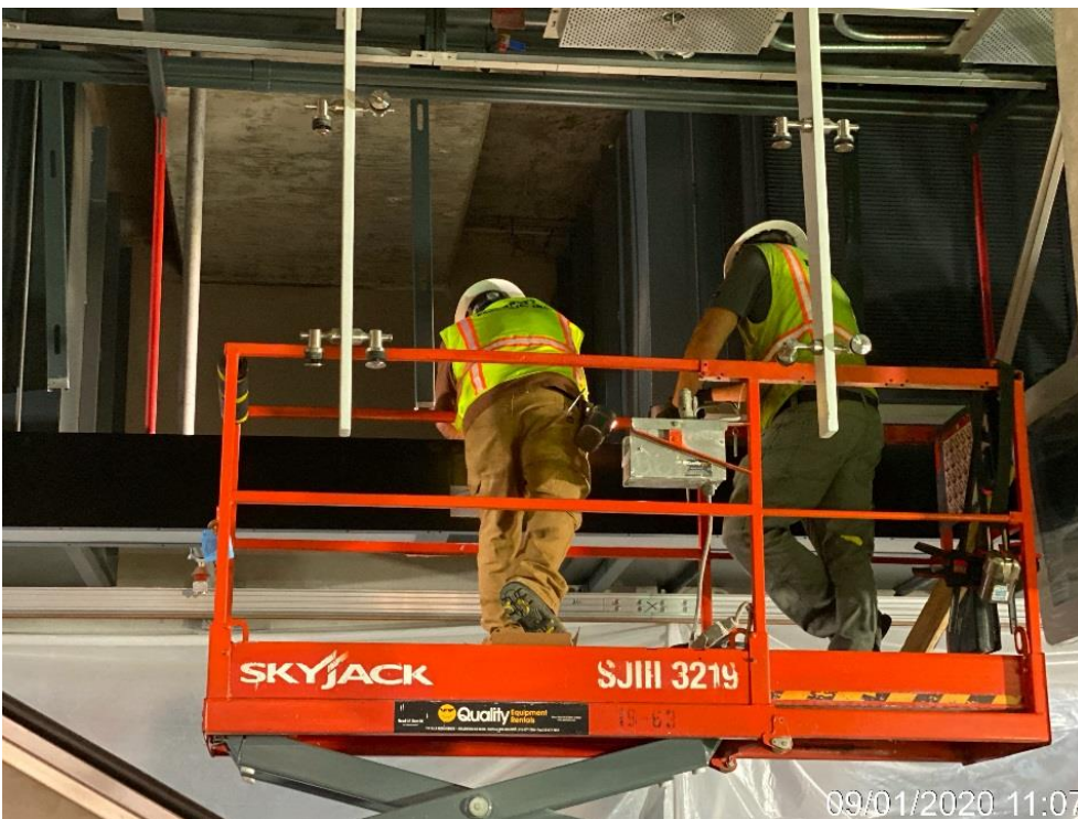
LEIMERT PARK STATION – Continue installing edge lights to the down stand support poles on both the north and southbound sides of the platform level.
