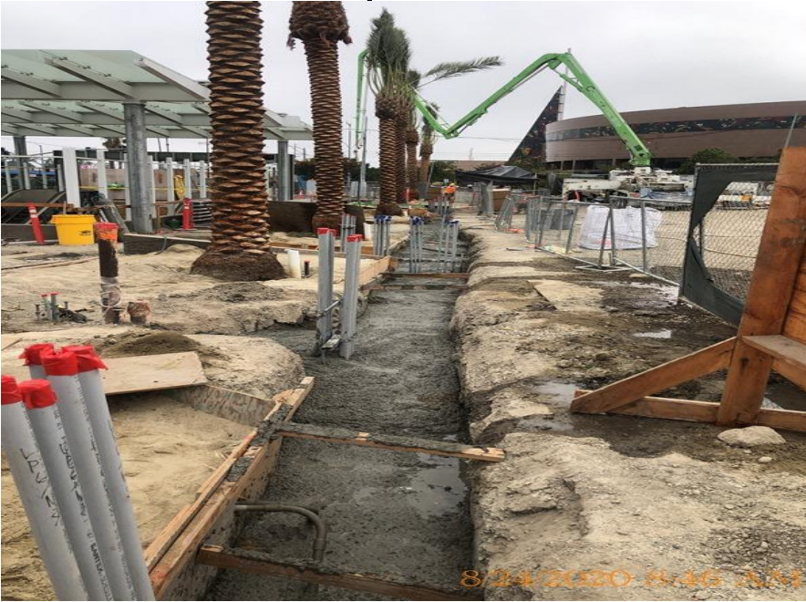
EXPO STATION – Placed and encased the landscape conduit duct bank trenches with concrete on the east side of the plaza level.
