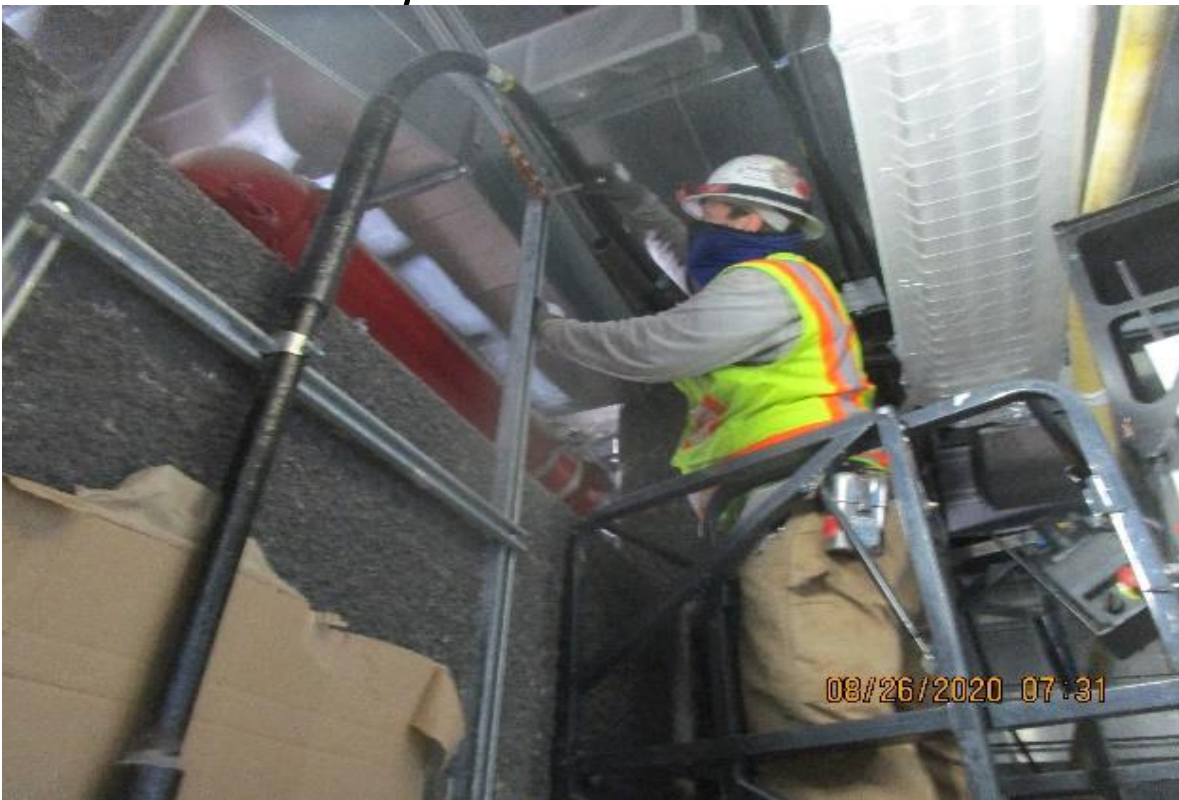
Crenshaw/Vernon – Vernon, EM Fan (N) C126, continued piping 2" FRP from LIP to EVF-6-302 factory instrument control PB
