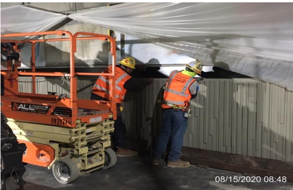
MLK STATION – WSCC crew prepping area and examining artwork at platform prior to applying fogging.
