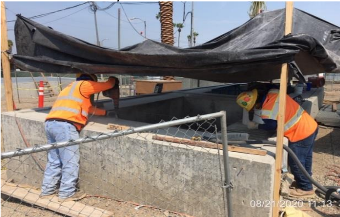
EXPO STATION SITE – Finishers chipping at vent shaft #3 to correct height for grating.
