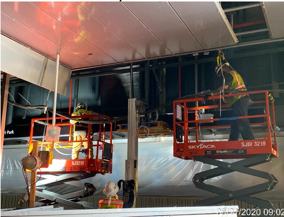
LEIMERT PARK STATION – Continue installing edge lights to the down stand support poles on the southbound side of the platform level.
