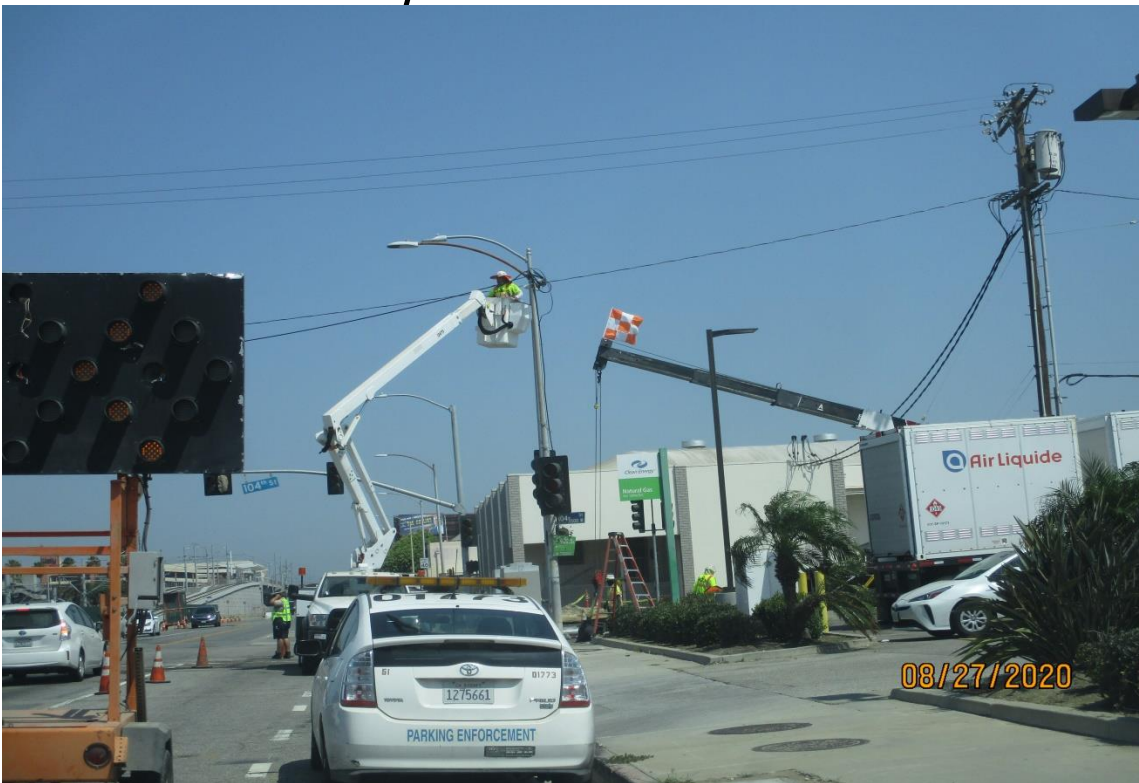
AVIATION/CENTURY- Lower a traffic signal pole at the SE corner of Aviation and 104th street.
