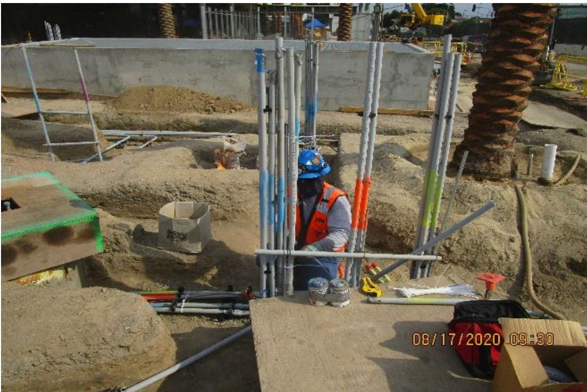
MLK STATION – MLK Plaza (SW) Continued underground electrical rough in (14) 1” PVC conduit to future PB for lighting circuits.
