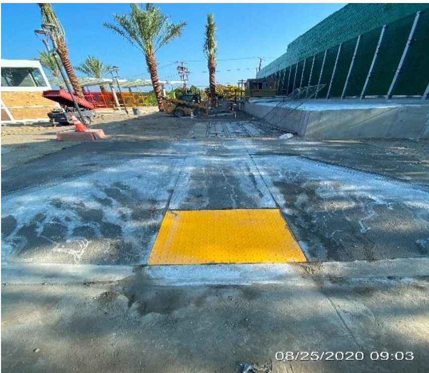
LEIMERT PARK STATION – Saw cut ADA ramp entrance (1 of 2) into the station plaza on the northeast corner of Crenshaw Blvd and 43rd Pl.
