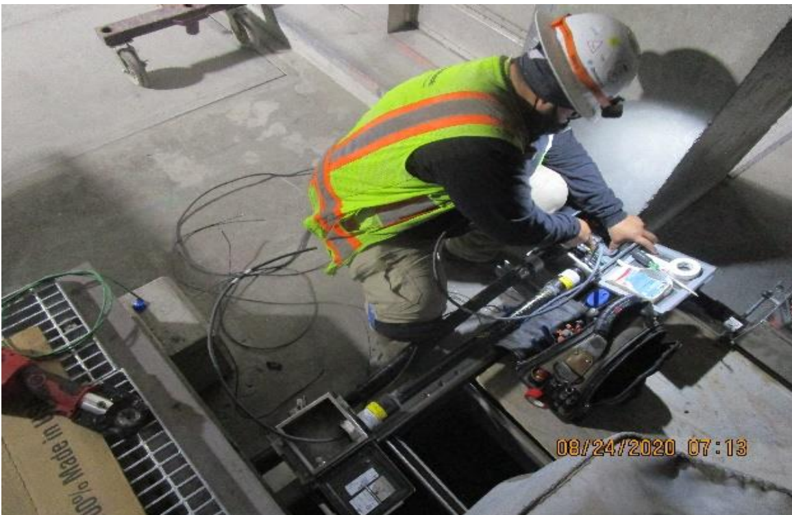
Crenshaw/Vernon – Vernon, Emergency fan south C102, continued TD's 6-301 identifying, labeling, dressing & terminating wiring.
