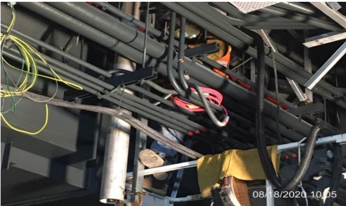
MLK STATION – WSCC ironworkers welding down stands on SB side of platform.
