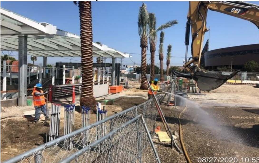
EXPO STATION – Backfilling and compacting trenches on the east side of the plaza level.
