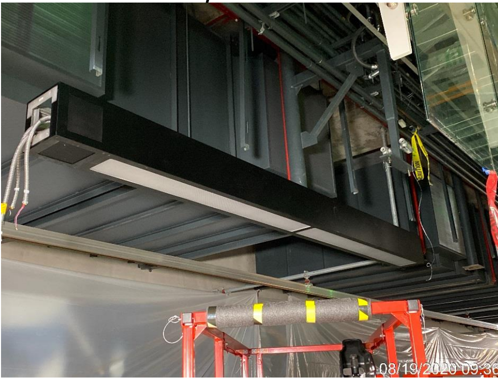
LEIMERT PARK STATION – Installing edge lights to the down stand support poles on the southbound side of the platform level.
