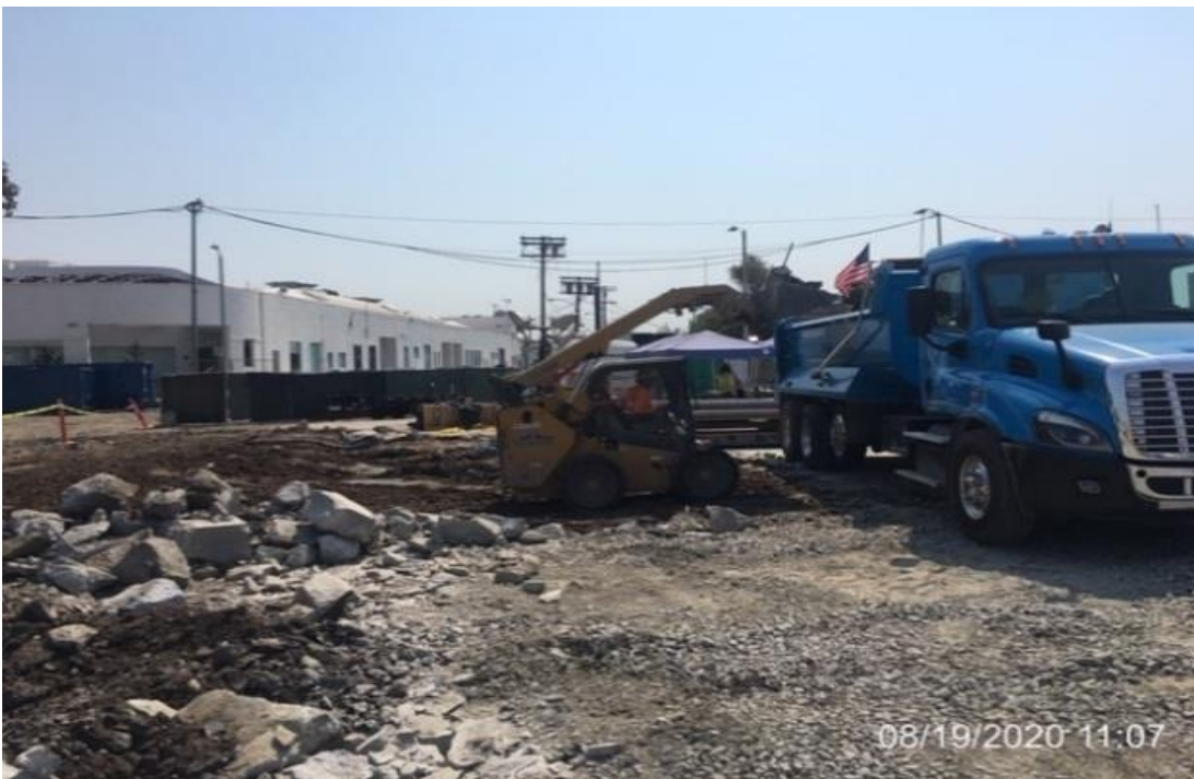
EXPO STATION – Continue demolishing/removing/hauling of existing concrete slab at the northern lot area.
