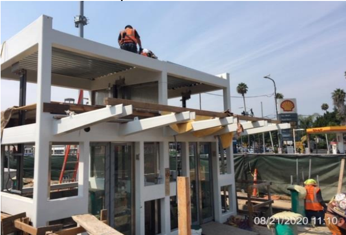
EXPO STATION – Continue installing metal roofing deck on top of Elevators 1&2 at the plaza level.
