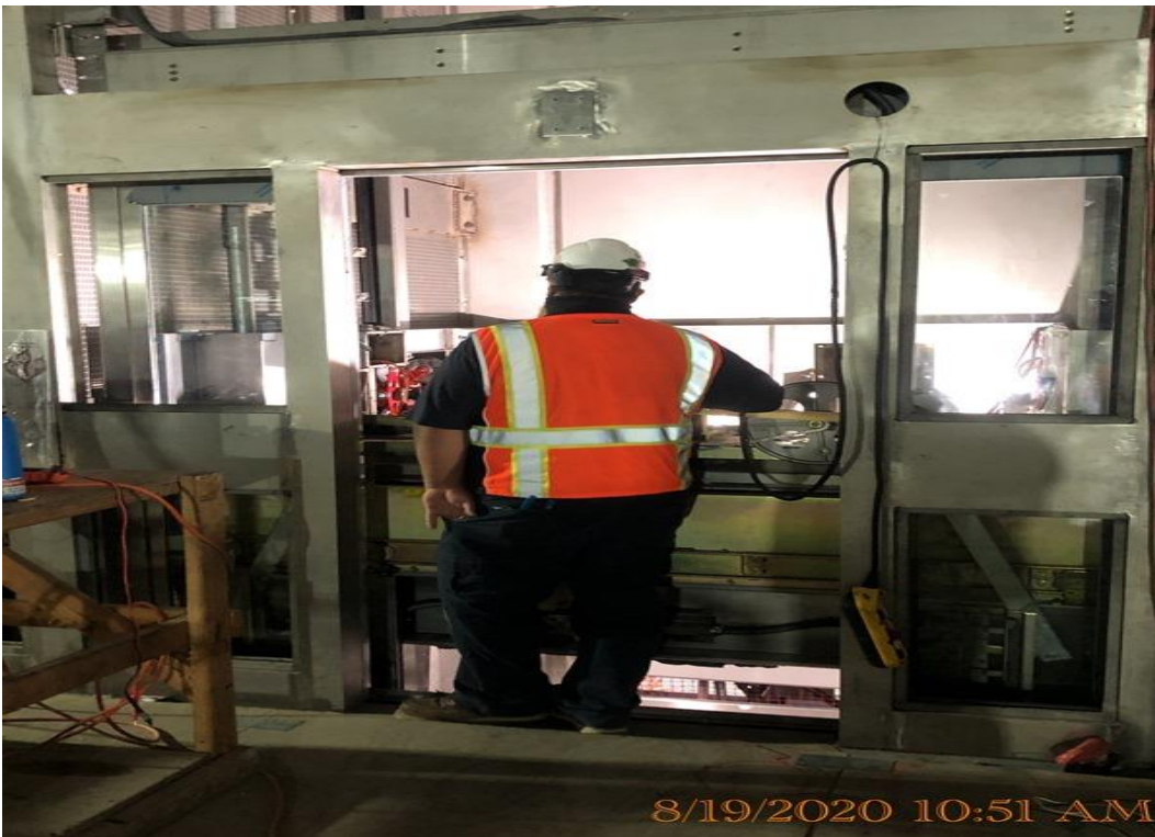
EXPO STATION – Continue final wiring and adjustments for all 4 Elevators at the concourse level.
