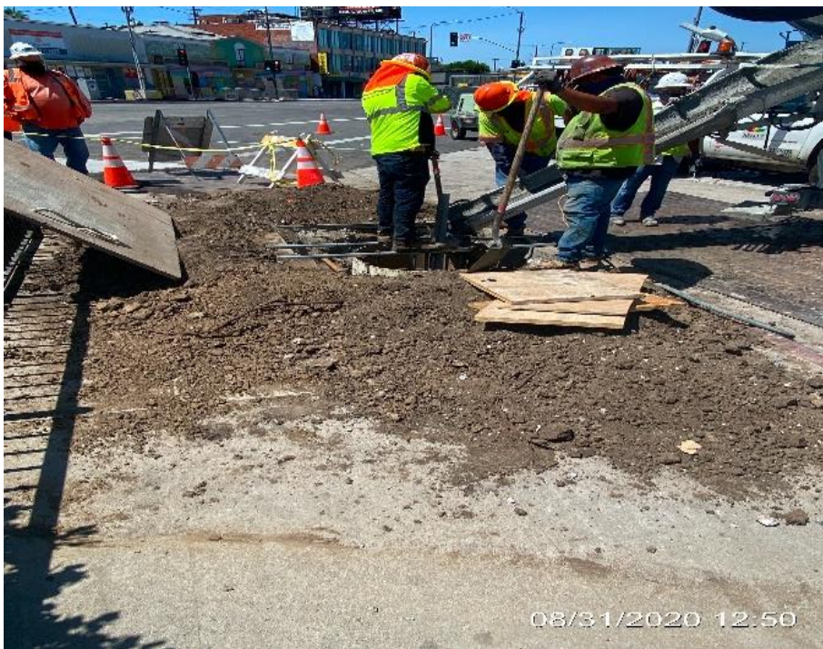
LEIMERT PARK STATION – Placing concrete for new street light pole foundation on the southeast corner of Crenshaw Blvd and 43rd Pl.
