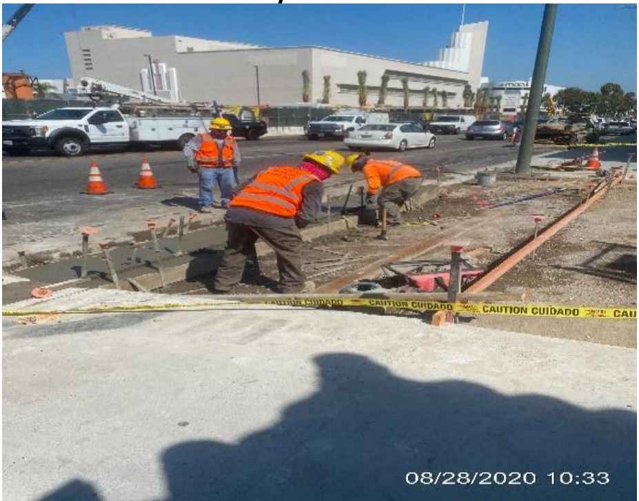
MLK STATION – Removing curb and gutter for restoration and placing concrete on northbound Crenshaw Blvd between Stocker St. and MLK Blvd.
