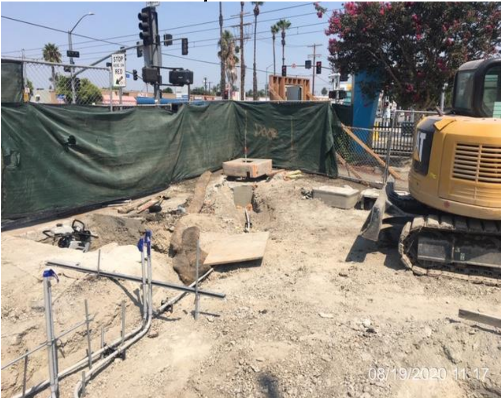
EXPO STATION – Excavating for the grand pylon foundation on the northwest corner of the plaza level.
