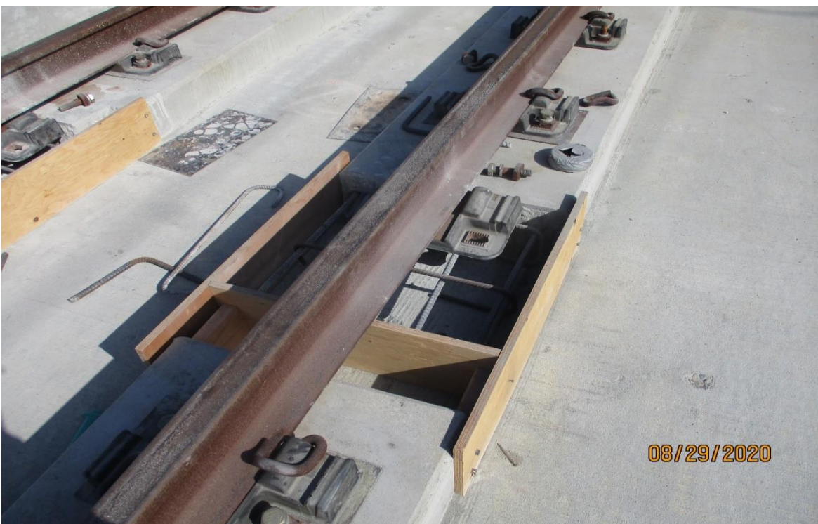
AVIATION/CENTURY- Drill and doweled rebar for the plinth repair on the Century bridge.
