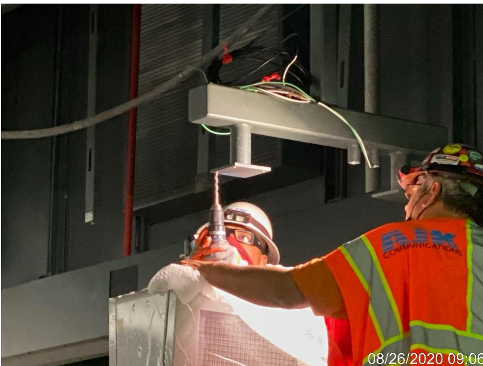
LEIMERT PARK STATION – Installing LCD/LED variable messaging sign monitors at the platform level.
