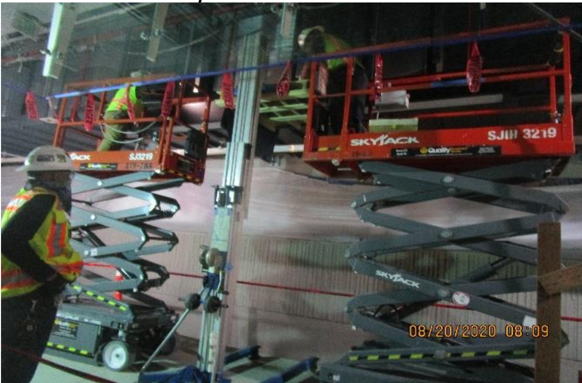
Crenshaw/Vernon – Vernon Platform, SB GL's 7-9/C, continued hanging & anchoring edge lighting to support post SB track #3.
