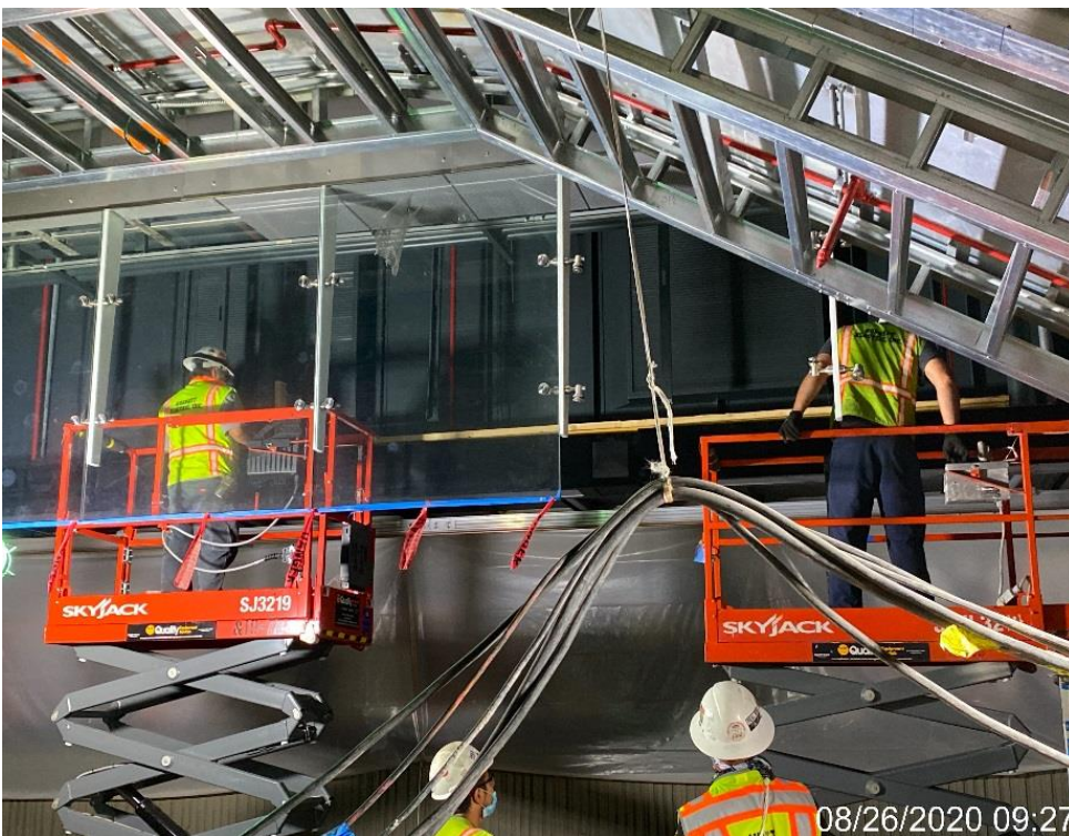
LEIMERT PARK STATION – Continue installing edge lights to the down stand support poles on the northbound side of the platform level.
