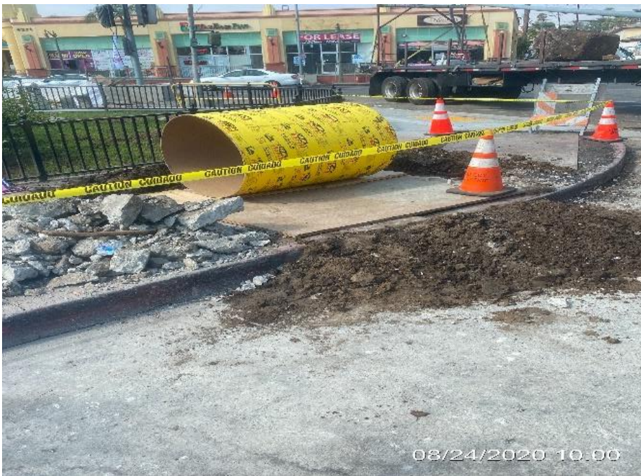
LEIMERT PARK STATION SITE – Preparing to form street light pole foundation on the southeast corner of Crenshaw Blvd and 43rd Pl.
