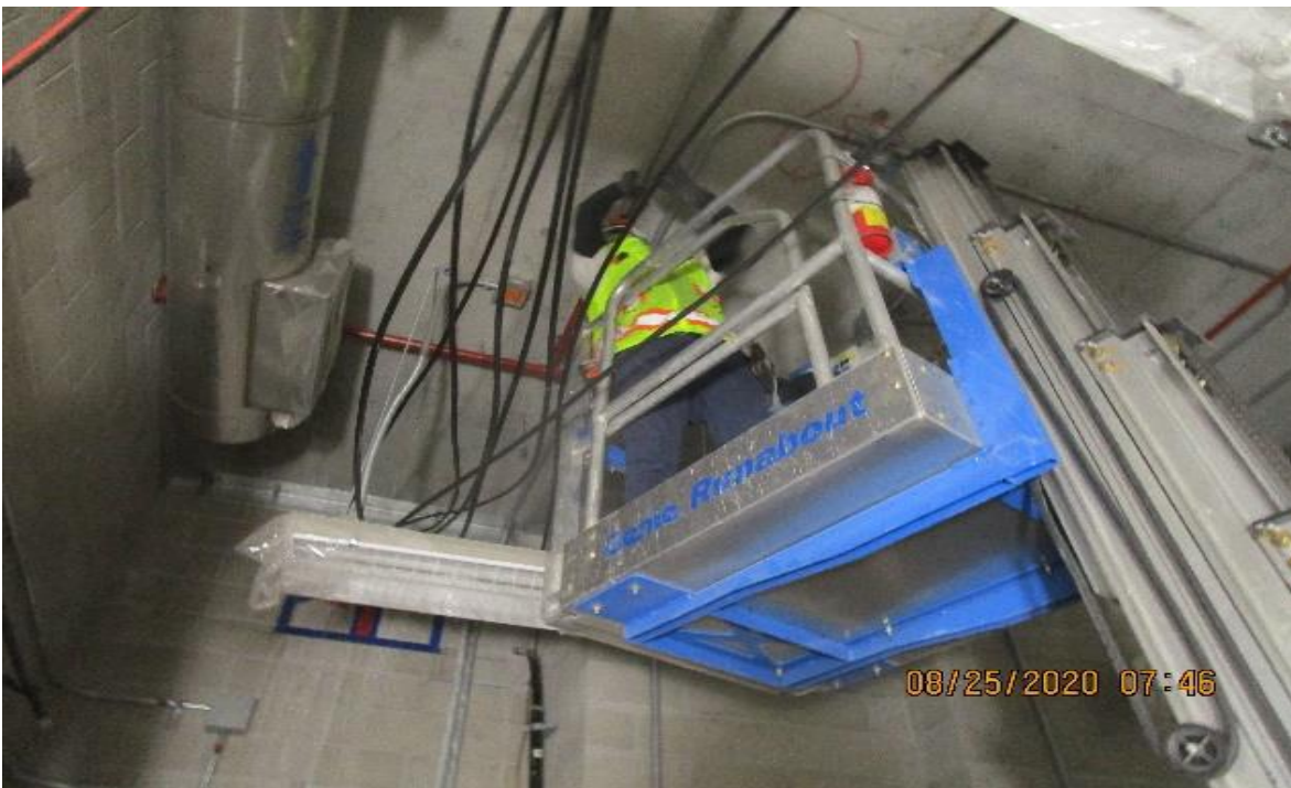
Crenshaw/Vernon – Vernon Battery room C113 (FA power supply) to TC&C C112 FATC continued supports & pipping 1” GRC.
