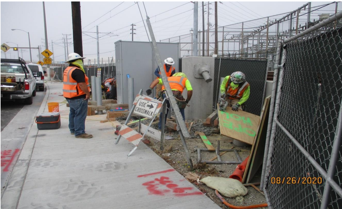
Hindry – Setting bollards around the meter pad and generator receptacle at the Hindry Station.
