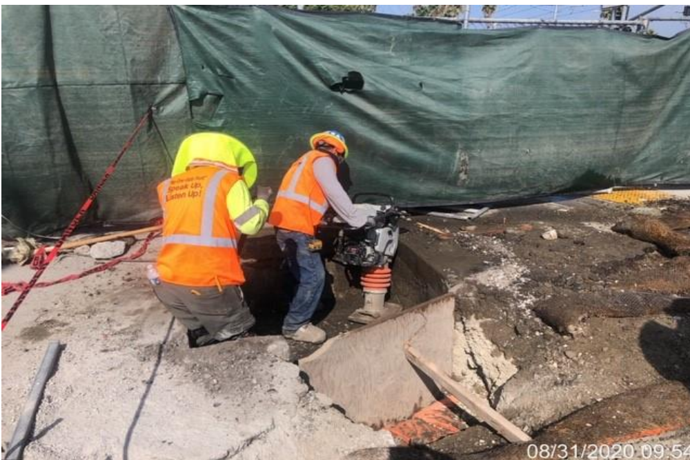
EXPO STATION SITE– Compacting grand pylon foundation on the northwest corner of the plaza level.
