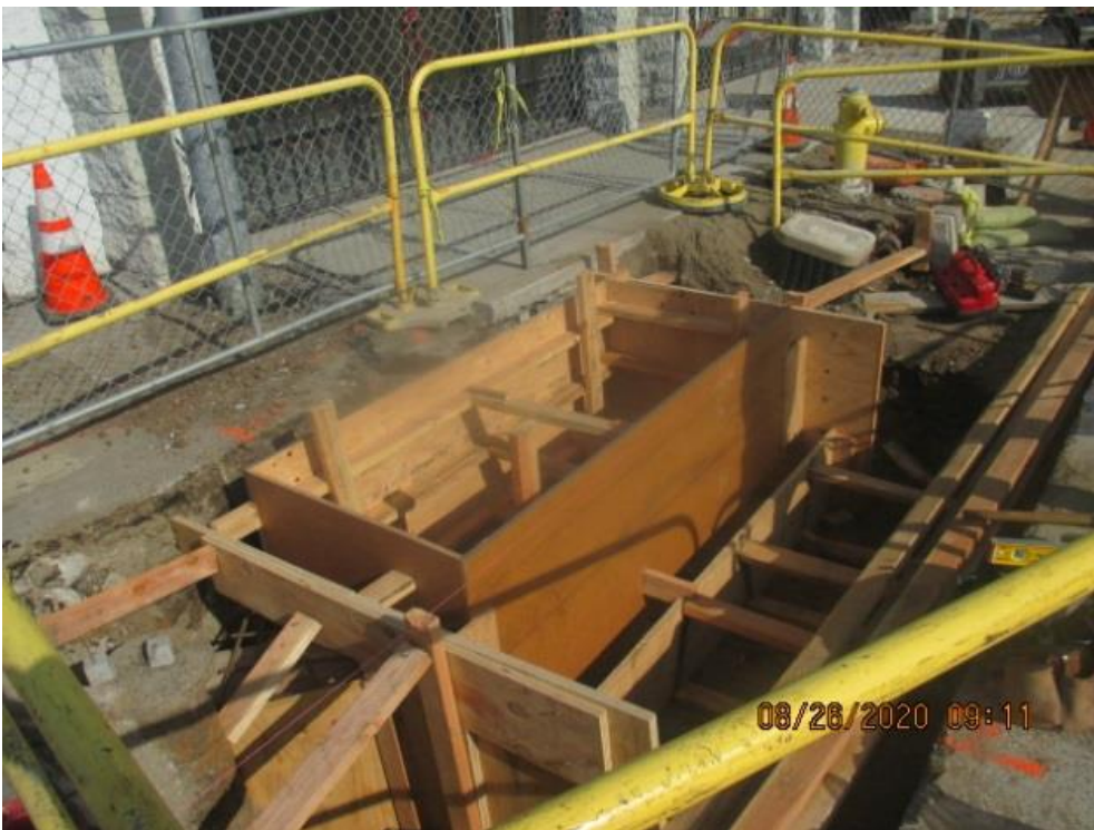
PARK MESA – Continue building stem wall forms for Catch Basin #30 on the northeast corner of Crenshaw Blvd and 67th St.
