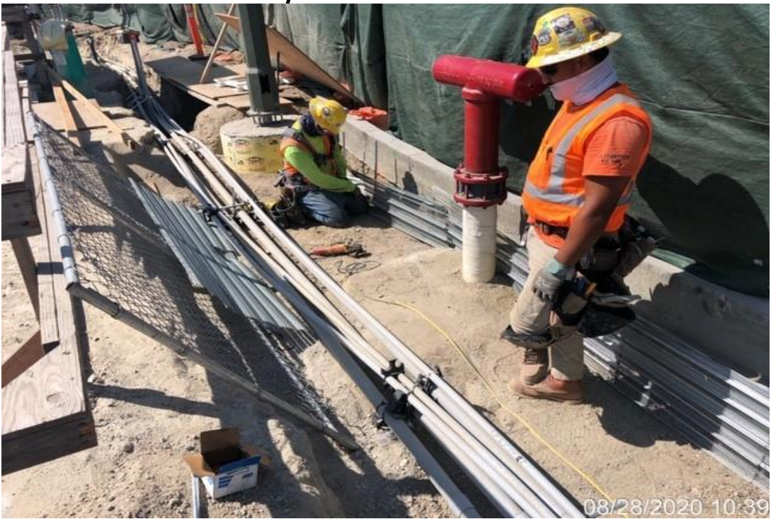
EXPO STATION – Continue installing conduit for landscape lighting on the west side trenches of the plaza level.
