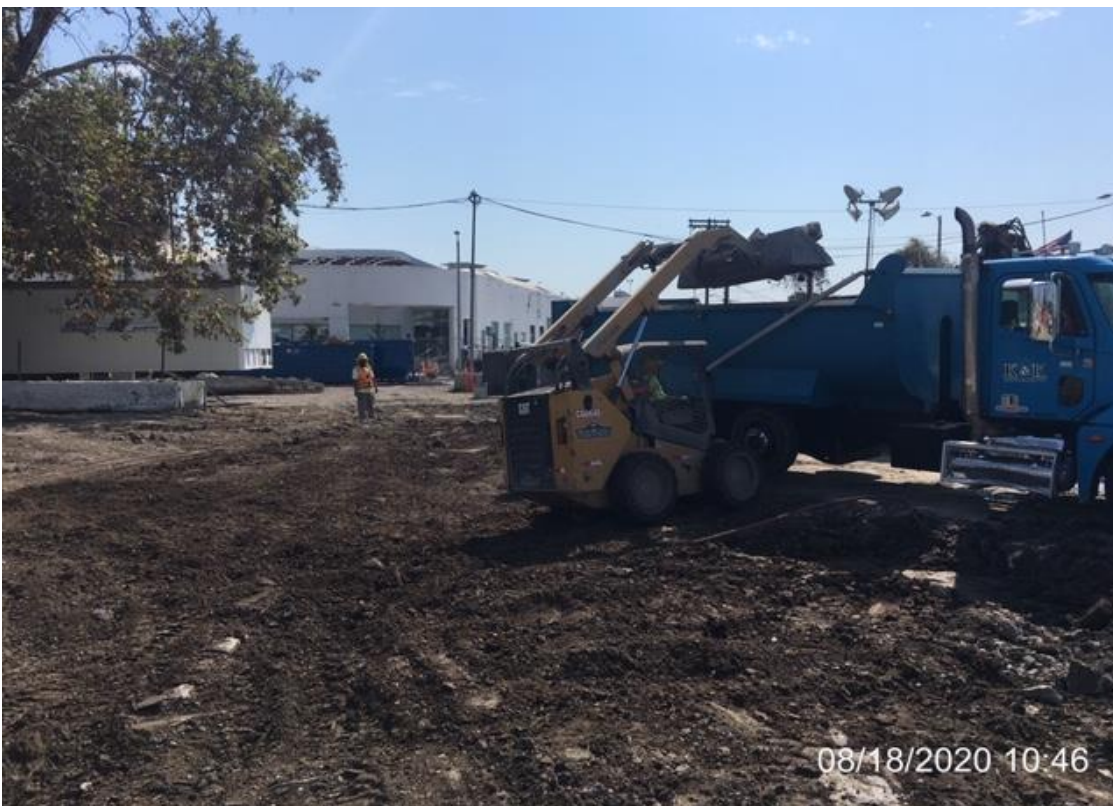
EXPO STATION– Keller water testing grout boxes and grouting at track level.
