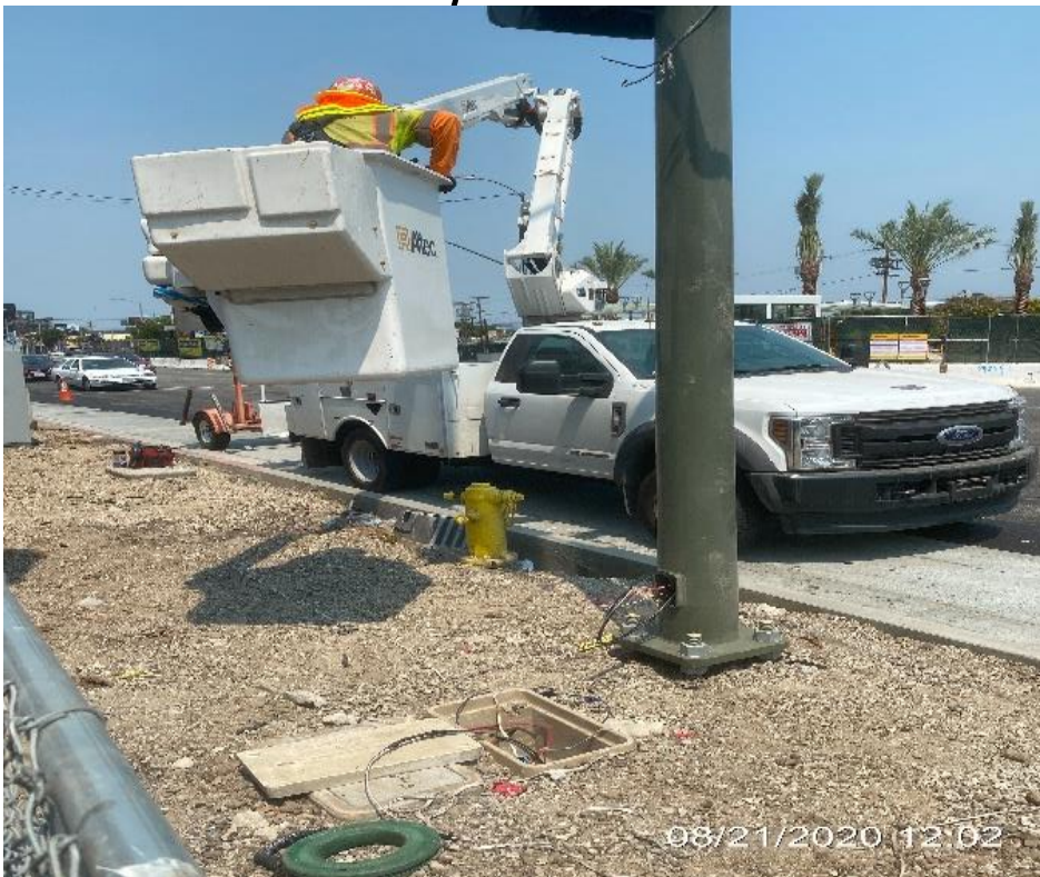
LEIMERT PARK STATION SITE – Installing overhead fixtures for the traffic signal light pole on southbound Crenshaw Blvd and 43rd St.
