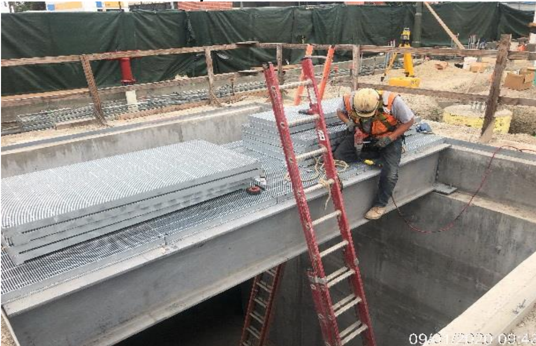
EXPO STATION – Anchoring grating panels to the Fresh Air Intake Shaft at the plaza.
