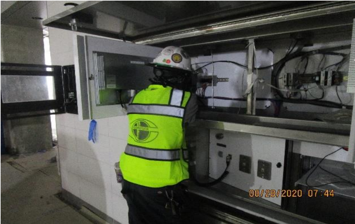
Crenshaw/Vernon – Vernon Paid Area C146, EMP Begin identifying, labeling & terminating #12 XHHW-2, Hot, Neutral & ground
