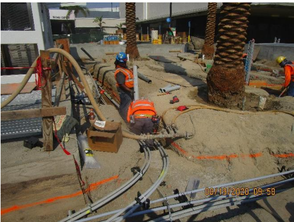
MLK STATION – Continue installing conduit for landscape lighting throughout the plaza level.
