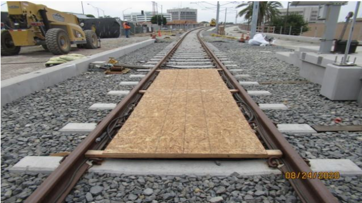
La Brea – LKC removed electrical track wiring on NB track at La Brea between STA 203+00 & 207+75 for HCC, WSCC to removal rails on NB track between these stations (looking north) Rework
