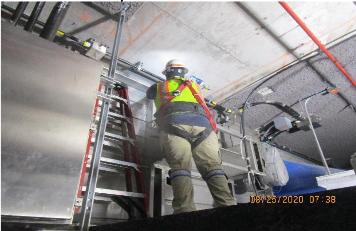
Crenshaw/Vernon – Vernon, Emergency fan south C102, continued BD's 6-101 identifying, labeling, dressing & terminating wiring.
