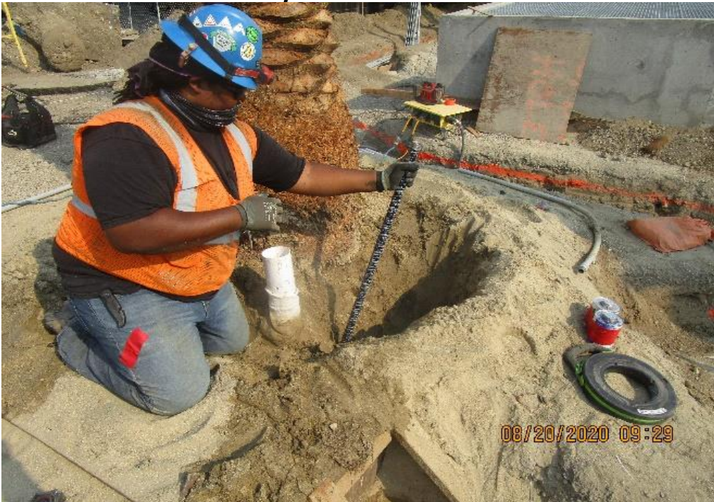
MLK STATION – Continue installing conduit for landscape lighting throughout the plaza level.
