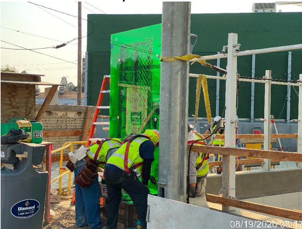
LEIMERT PARK STATION – Installing art glass panels around the main entrance canopy structure at the plaza level.
