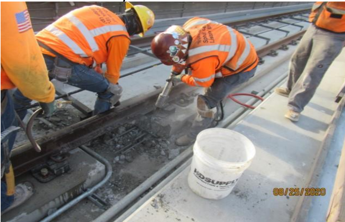
AVIATION/CENTURY- WSCC control demoing end of plinth on SB track Century/Aviation bridge for NCR-A 111 case 4 Rework.
