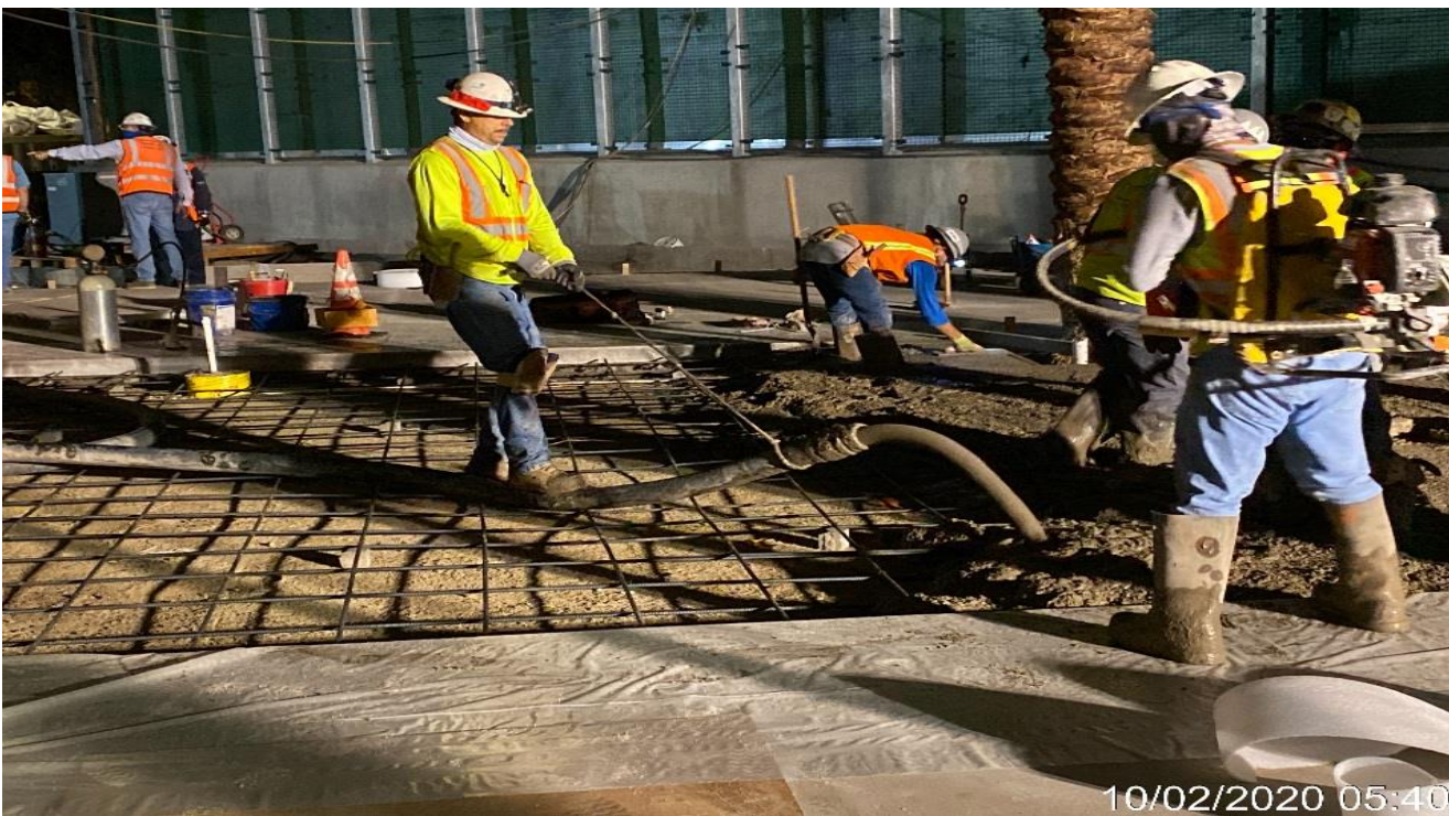
LEIMERT PARK STATION SITE – Continue placing concrete for the architectural topping slab throughout the plaza level.
