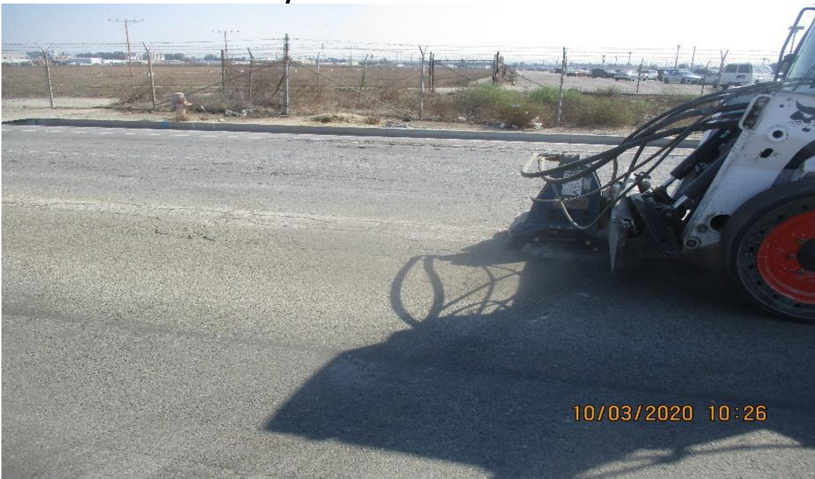
AVIATION/CENTURY- SCI Removed all stripping on S/B Aviation from 104th to 111th ST.
