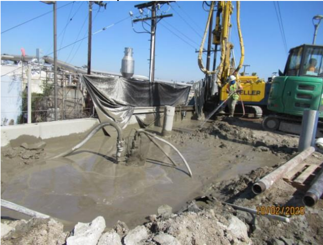
La Brea – MSE wall 202 La Brea SB track STA 207+50 on-going jet grout operation (looking northwest) Rework NCR B-089.
