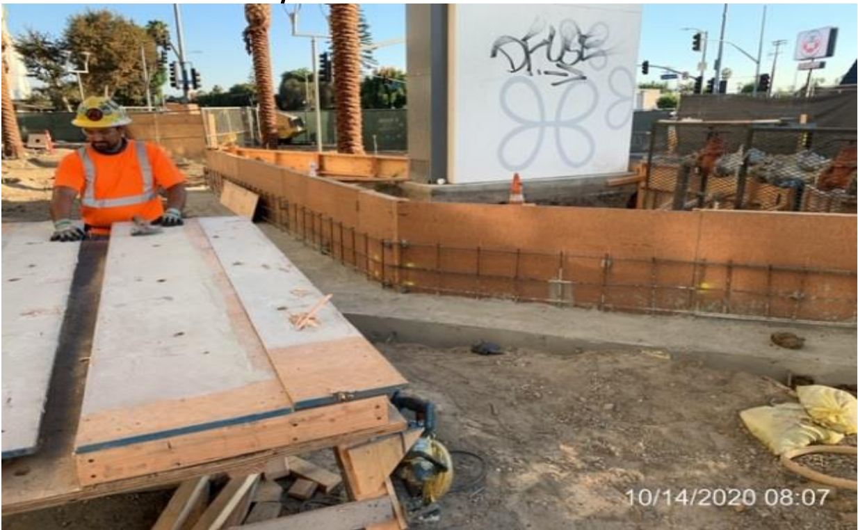
MLK STATION – Continue building formwork for the north end planter wall at the plaza level.
