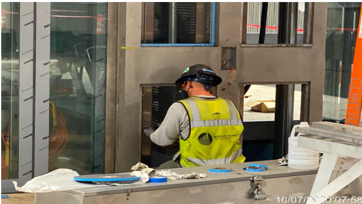
LEIMERT PARK STATION – Continue installing glass tracks for Elevators 3&4 at the platform level.
