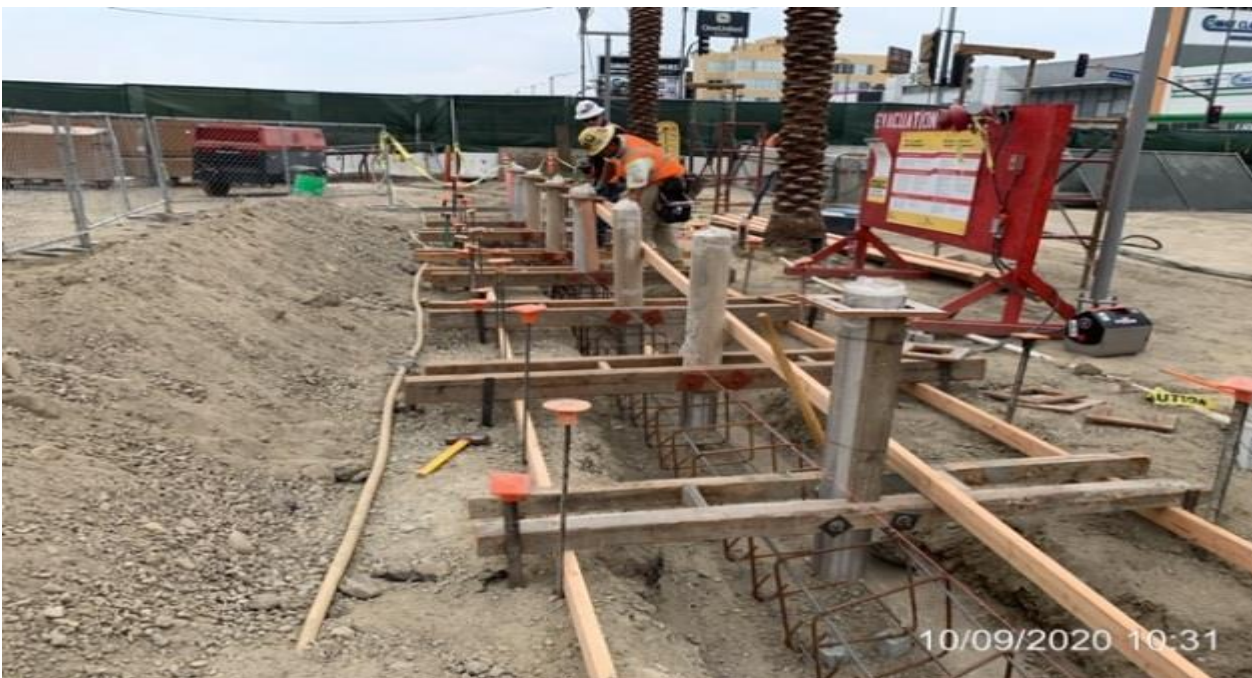
EXPO STATION - Building formwork and setting the east side bollard foundations at the plaza level.
