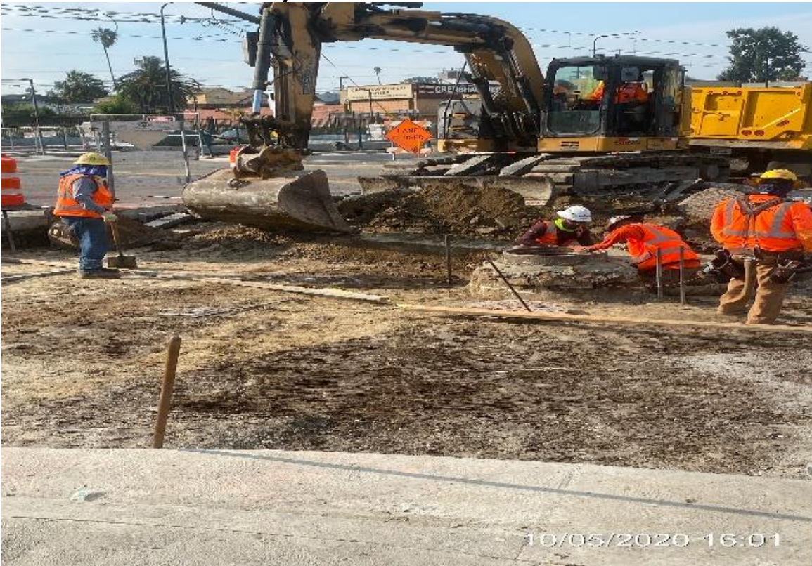
PARK MESA – Sacking and patching sewer maintenance hole on northbound Crenshaw Blvd and 52nd St.
