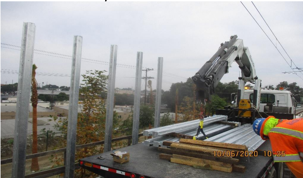
La Brea – Ace Fence placing extra strength fence post at wall 202 at La Brea Sta.
