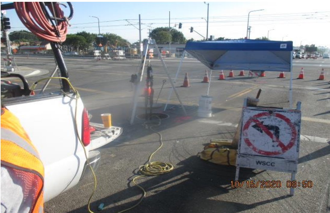
PARK MESA – Sacking and patching and installing ladder rungs to Manhole #12 and #16 on southbound Crenshaw Blvd and Slauson Ave.
