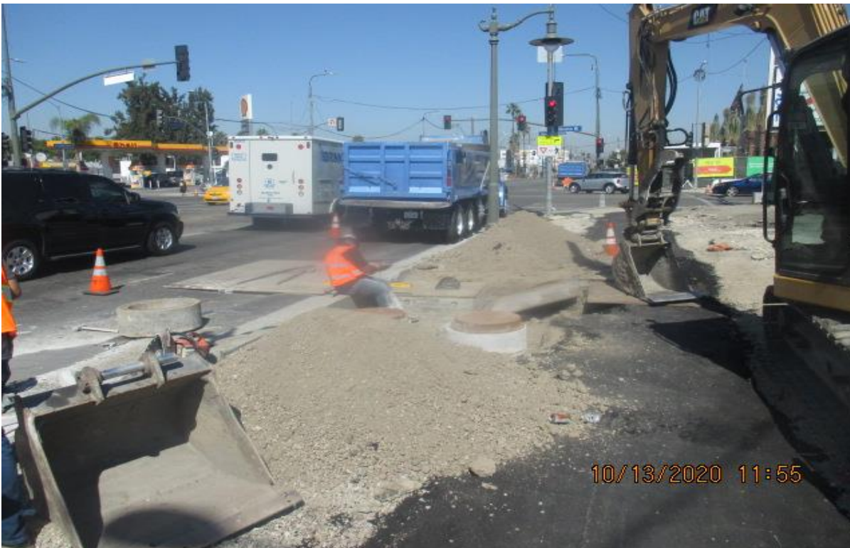
EXPO STATION – Setting final elevations for access covers along northbound Crenshaw Blvd south of Obama Blvd.
