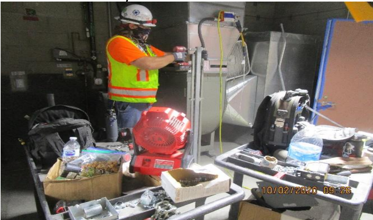
MLK STATION – MLK Concourse, Mechanical room (N) C128 Continued 1” GRC piping exhaust & supply fan limit switches.
