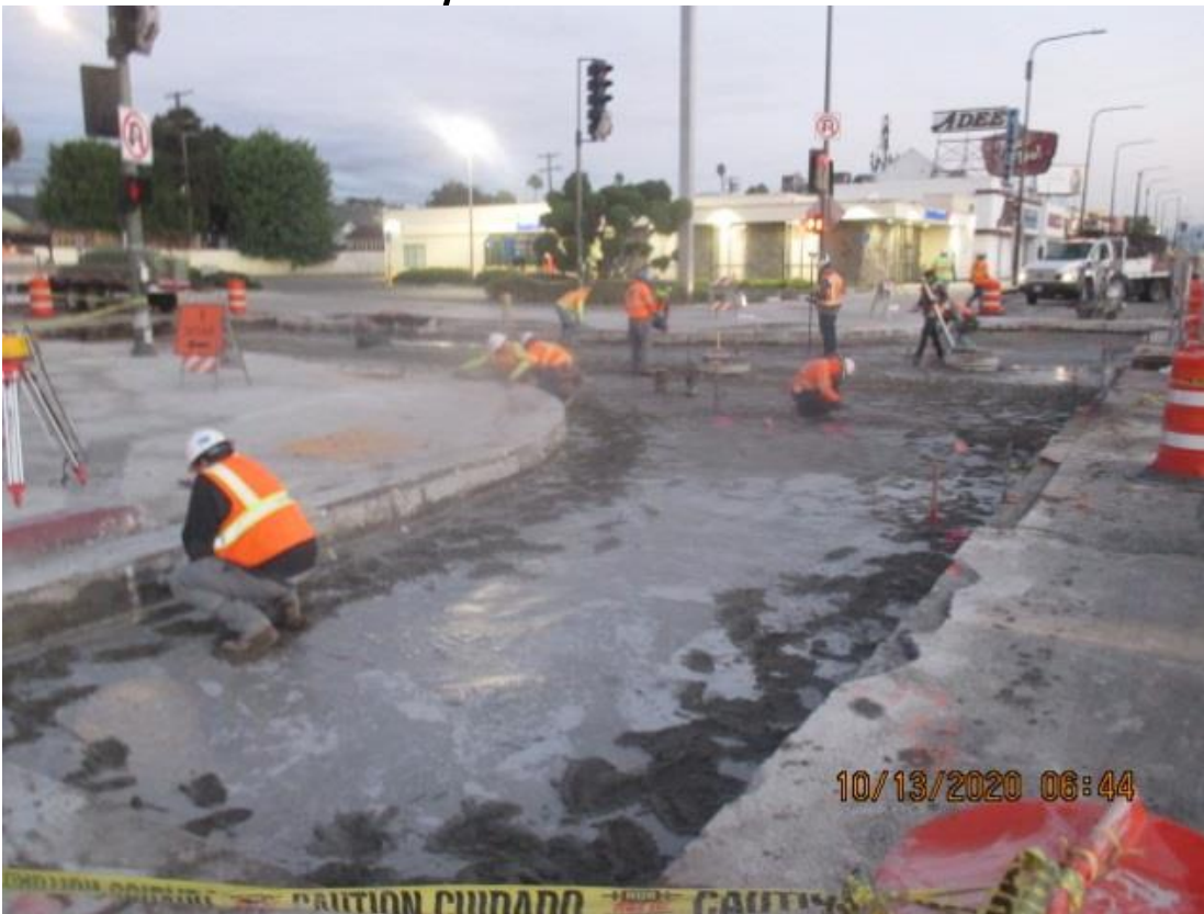
PARK MESA – Continue building formwork and placing slurry on the north and southbound lanes for restoration at the intersection of Crenshaw Blvd and 57th St.
