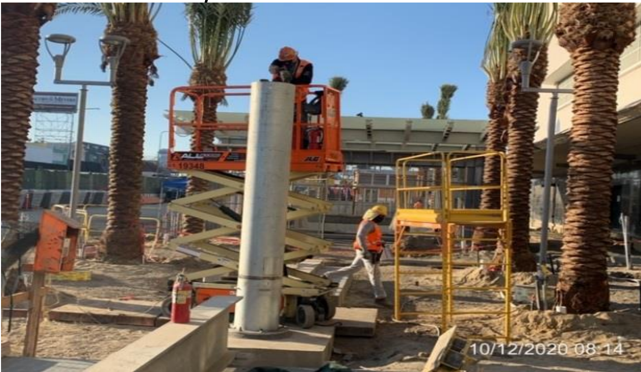
MLK STATION – Welding pipe clamps to the north and south plumbing vent stack at the plaza level.
