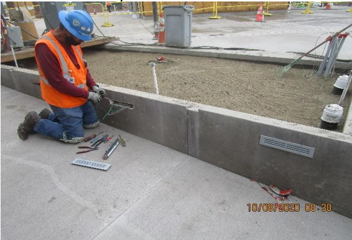
Crenshaw/Vernon – Vernon Plaza, began installing foreign (made in chine) recessed ramp & stair lighting without UL listing.
