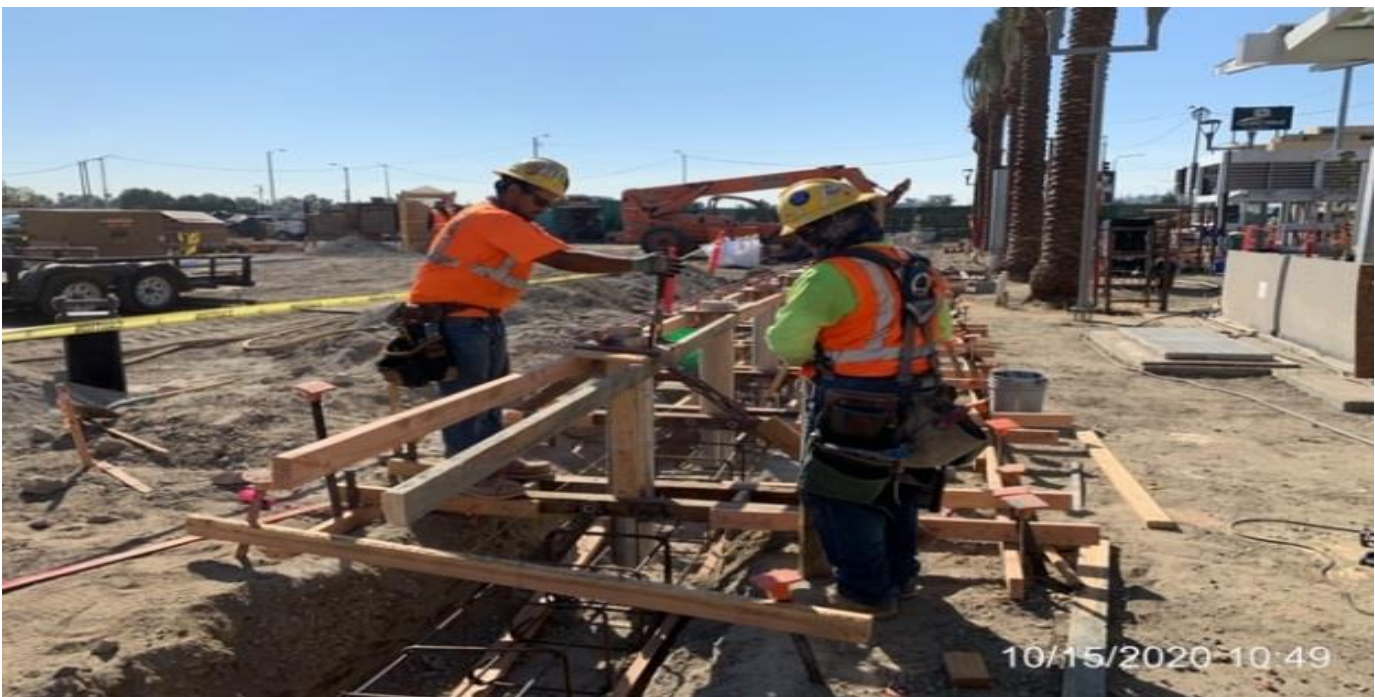
EXPO STATION – Continue building formwork and setting the east side bollard foundations at the plaza level.
