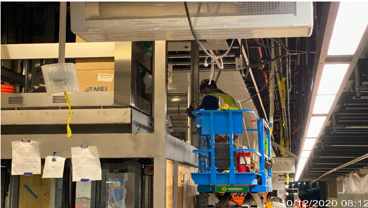
LEIMERT PARK STATION – Continue installing glass tracks for Elevators 3&4 at the platform level.
