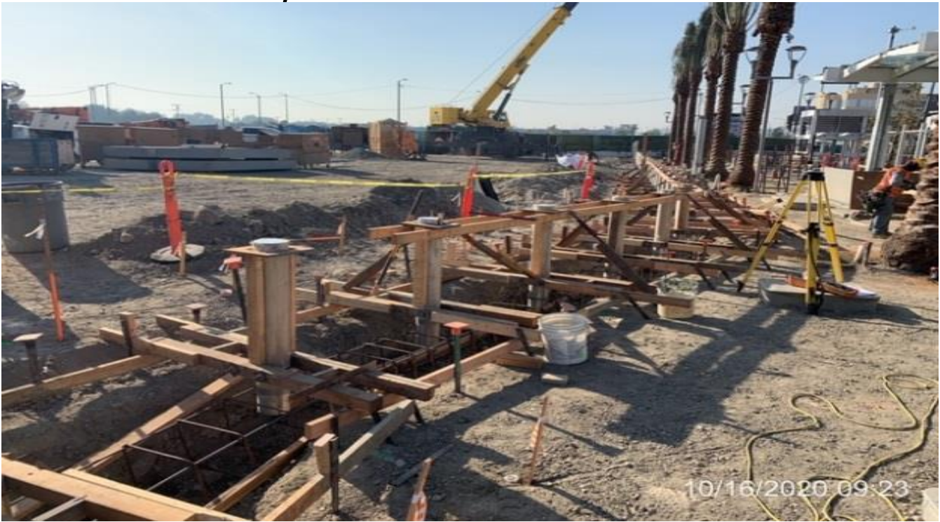
EXPO STATION – Continue building formwork and setting the east side bollard foundations at the plaza level.
