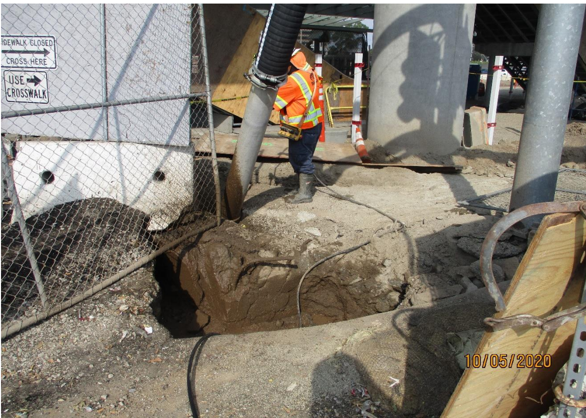
AVIATION/CENTURY- Daylighting a foundation in conflict with the traffic signal conduit on the NEC of Century and Aviation.
