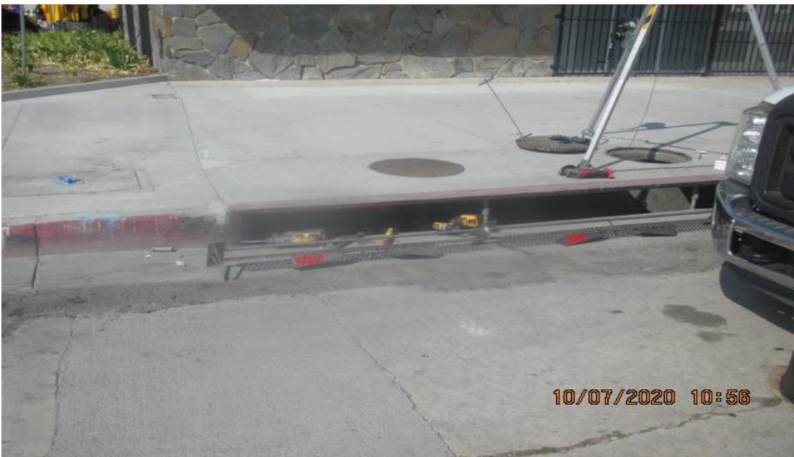
PARK MESA – Installing protective gratings for opening of Catch Basin #33 on Crenshaw Blvd and 57th St.
