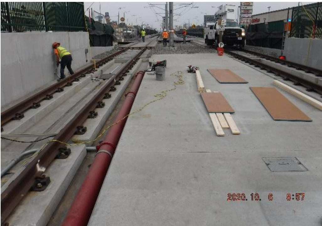
59 th Street – STA 316+00 TK#3/SB looking north – form work and conduits set-up for traffic control loops, north end of UG3 at 59th St at grade Xing
