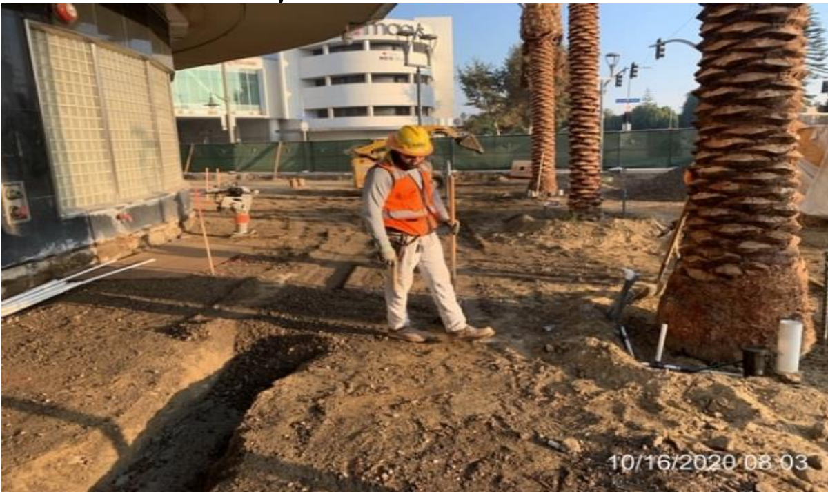
MLK STATION – Continue installing root watering system and valves for the palm trees at the plaza level.
