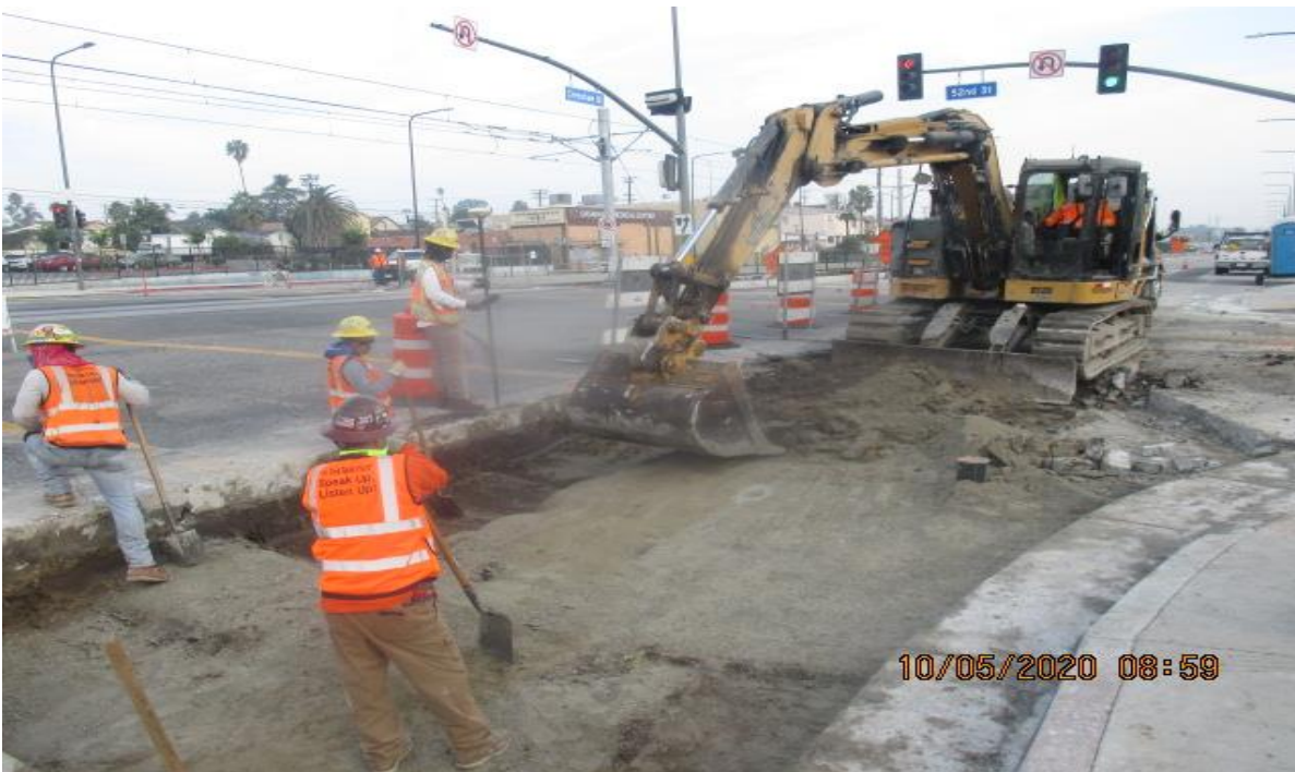
PARK MESA – Excavating northbound lanes for restoration on Crenshaw Blvd and 52nd St.
