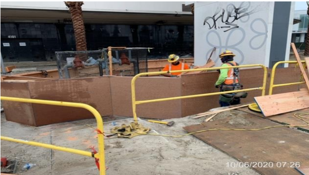
MLK STATION – Building formwork for the north end planter wall at the plaza level.
