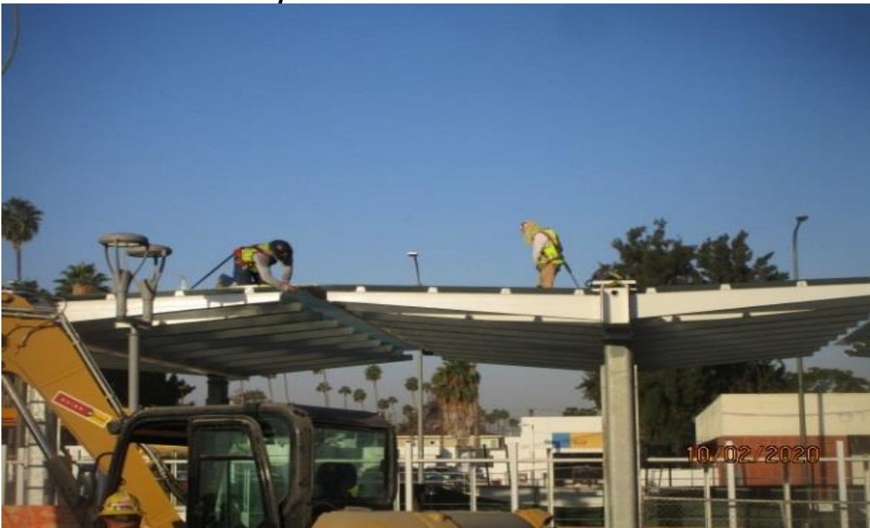
EXPO STATION – Caulking and sealing expansion joints for the glass roof of the main entrance canopy at the plaza level.
