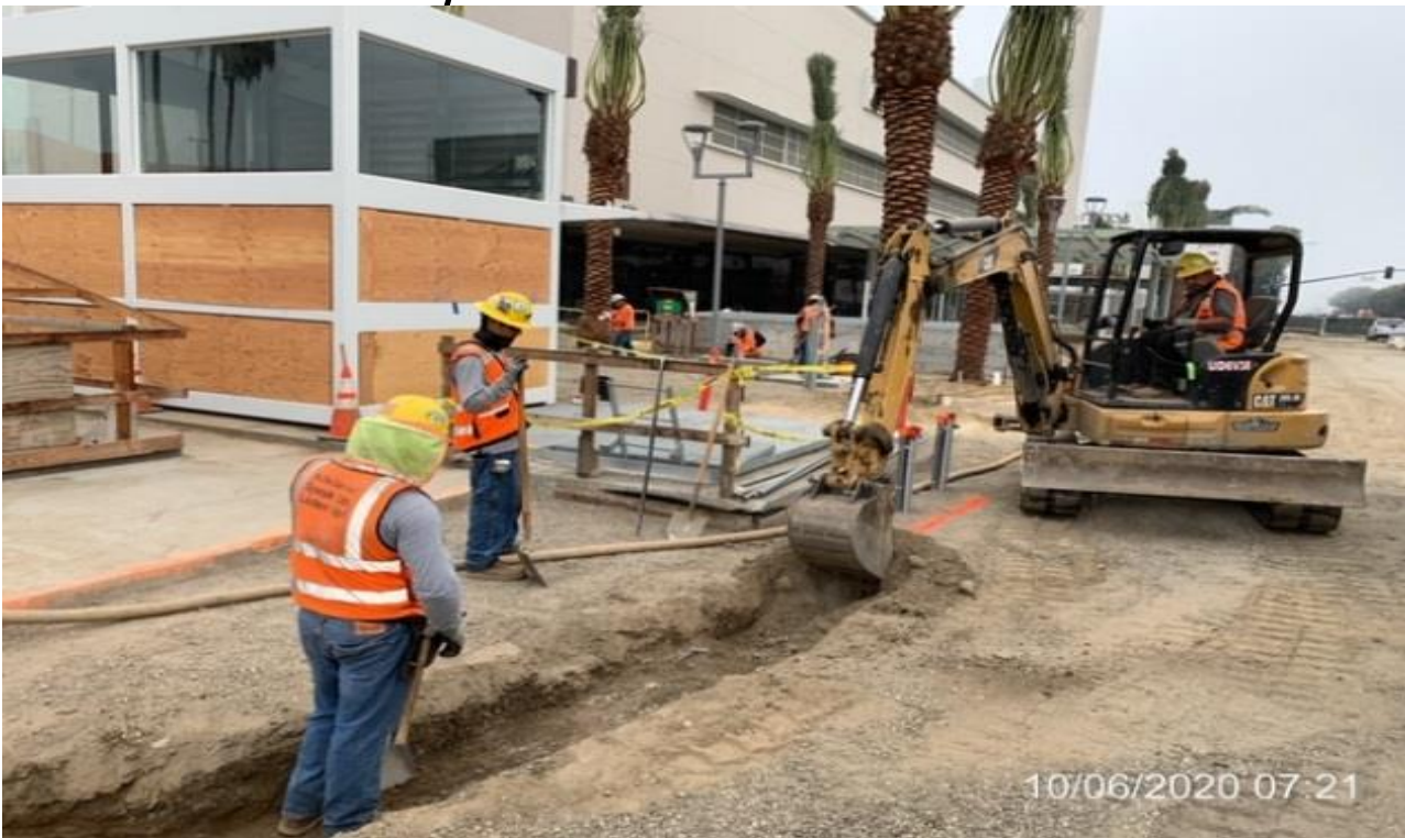
MLK STATION – Excavating for CCTV conduit for the pedestrian light poles at the plaza level.
