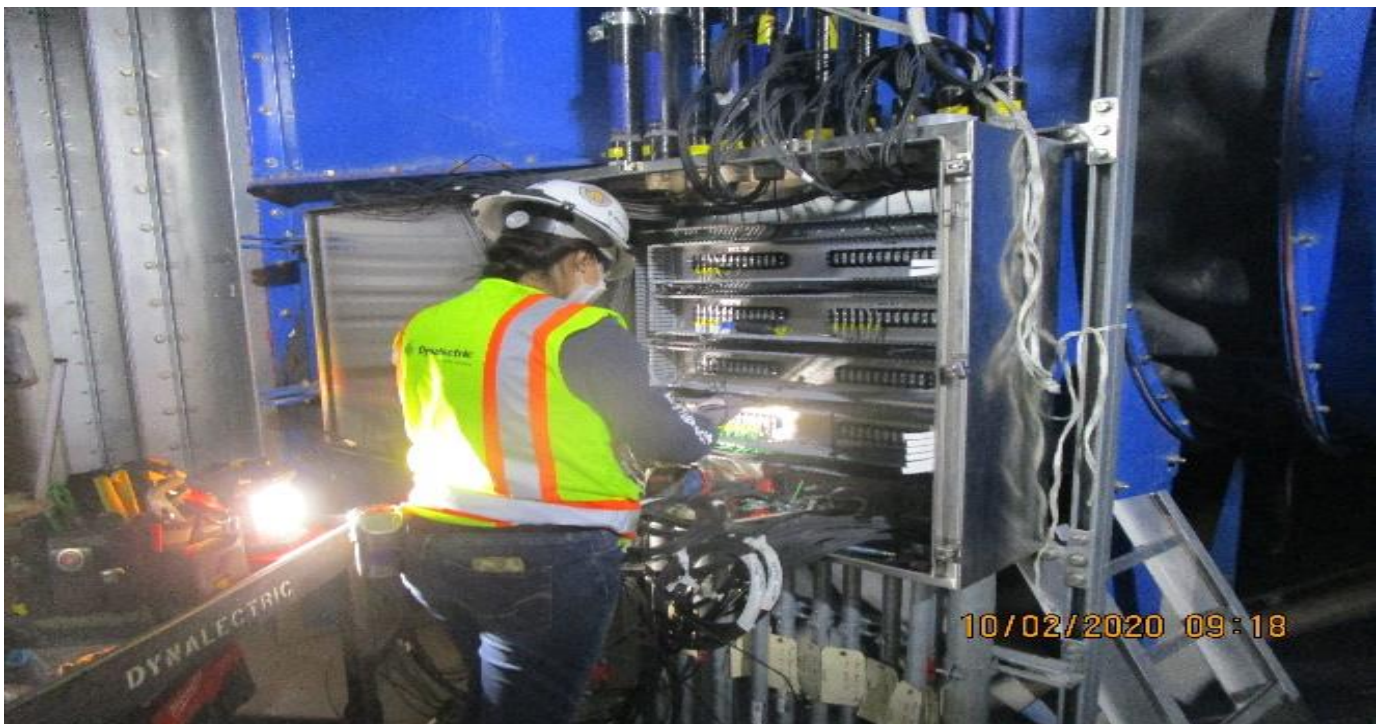
MLK STATION – MLK EM Fan (S) C102, EVF-7-121, continued, terminating power, controls for OTED, BD, TFD & TD's.
