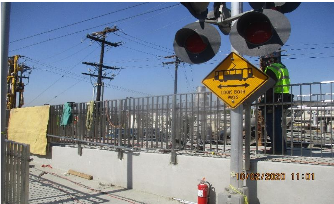
La Brea – McMahan Welding and placing handrails at S/La Brea handy capped ramps.
