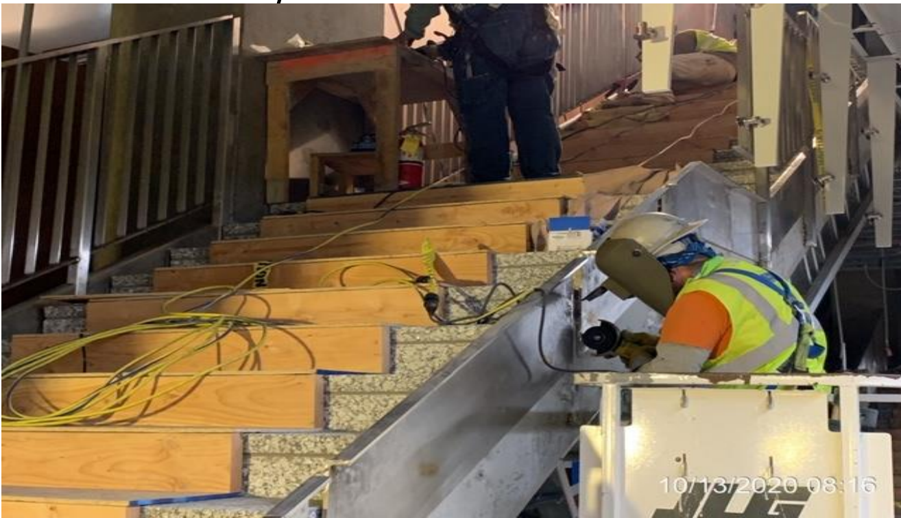
MLK STATION – Continue welding and installing guardrails to Staircase #2 from concourse to platform level.
