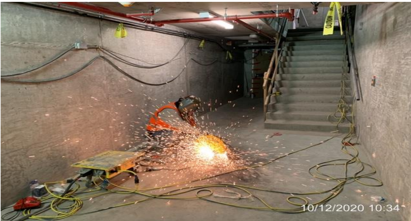
EXPO STATION – Continue installing grid support system and base plates for the mosaic art wall at the concourse level.
