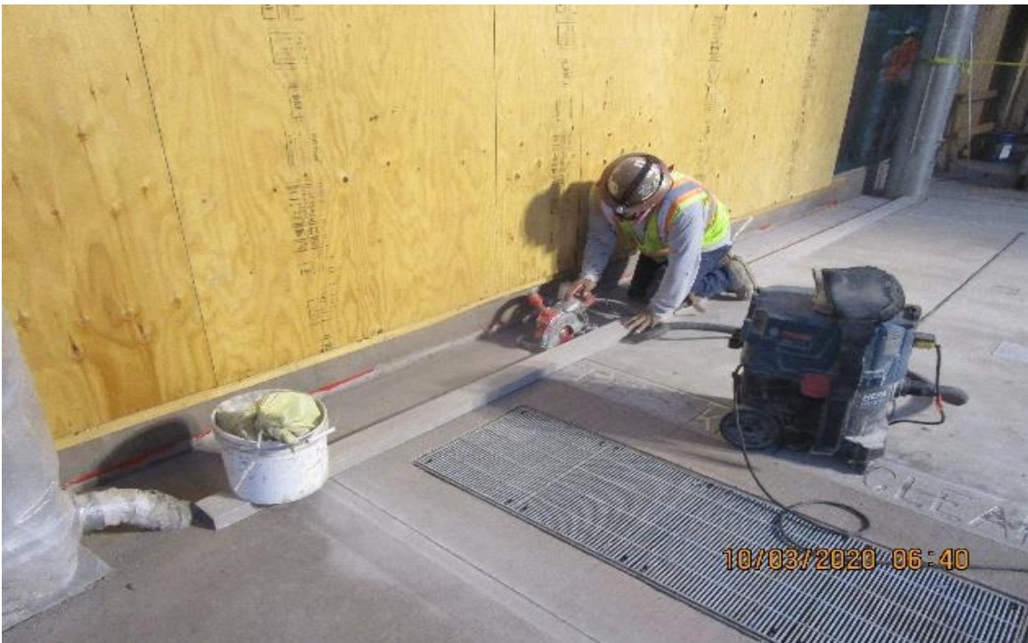
Crenshaw/Vernon – Vernon Plaza level, continued saw cutting 3/16” expansion joints at architectural concrete & stripping of form work
