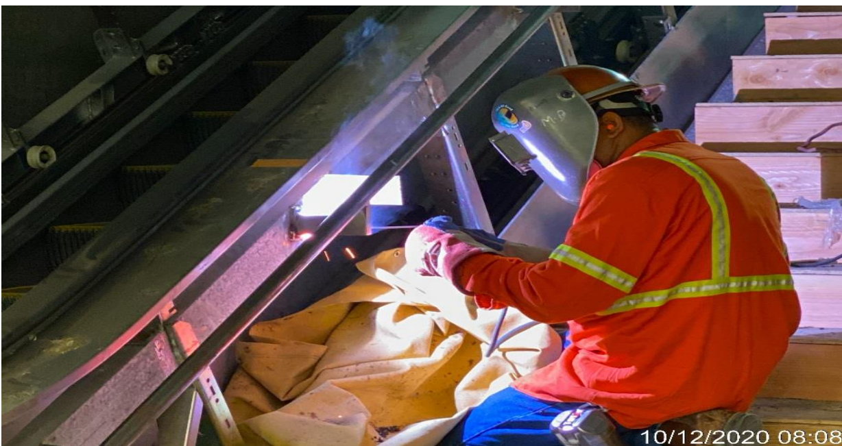
LEIMERT PARK STATION – Continue installing brackets for handrails at Staircase #2 from intermediate landing to platform level.
