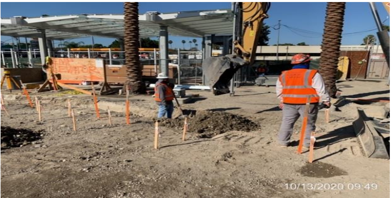
EXPO STATION – Continue building formwork, setting, and excavating for the east side bollard foundations at the plaza level.
