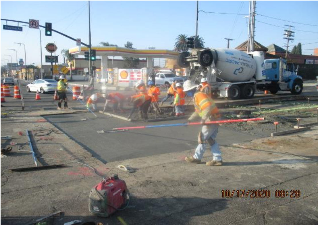
PARK MESA – Continue placing rebar and concrete over north and southbound lanes on Crenshaw Blvd and Slauson Ave.
