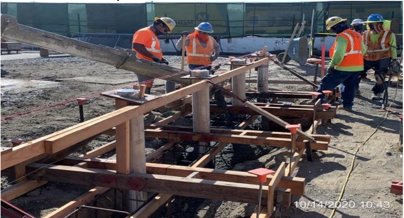
EXPO STATION – Setting rebar and placing concrete for the east side bollard foundations at the plaza level.
