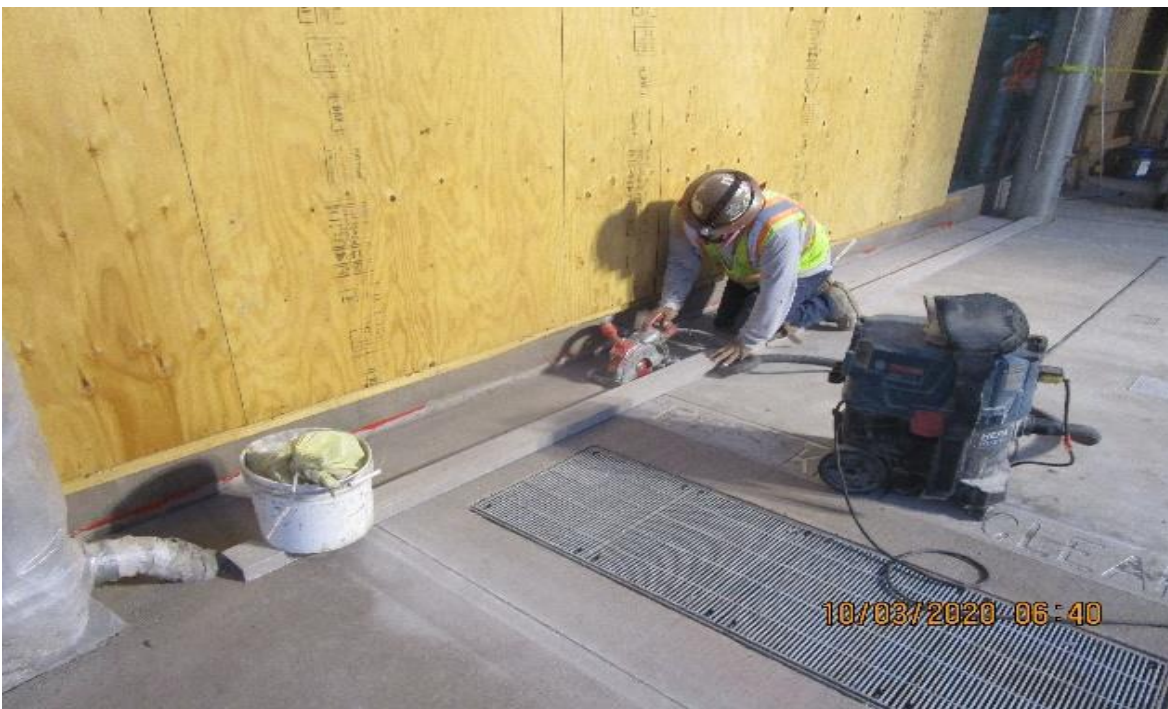
LEIMERT PARK STATION – Continue saw cutting control joints for the architectural topping slab throughout the plaza level.
