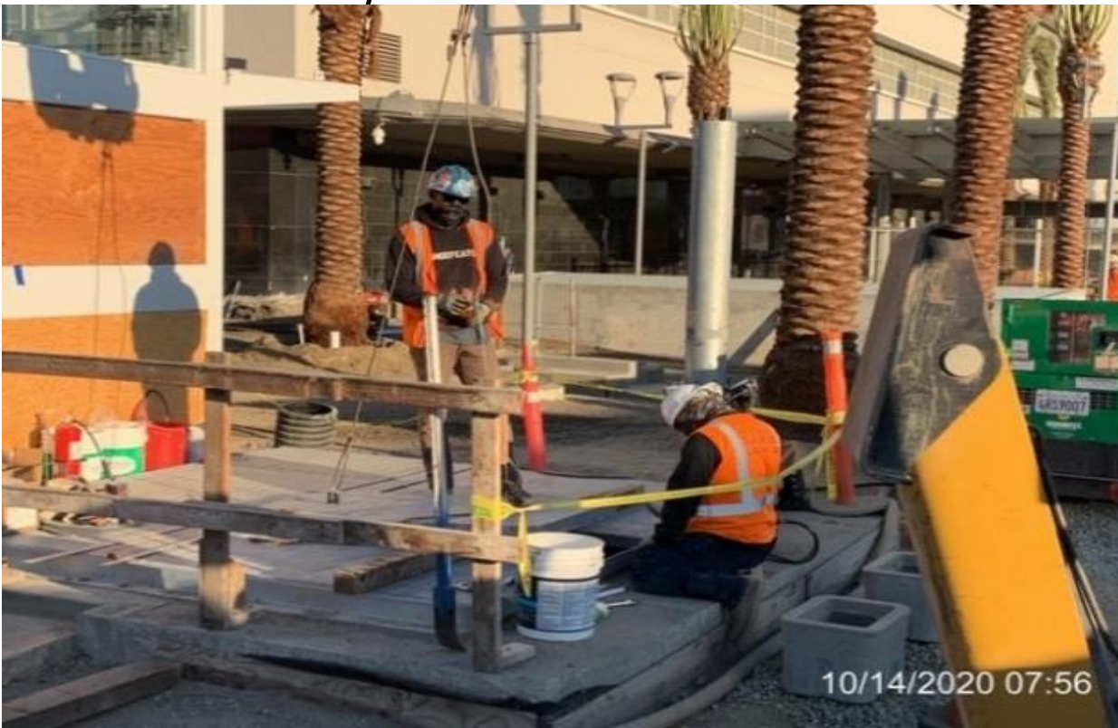
MLK STATION – Anchoring and aligning grating to Fresh Air Intake #1 at the plaza level.
