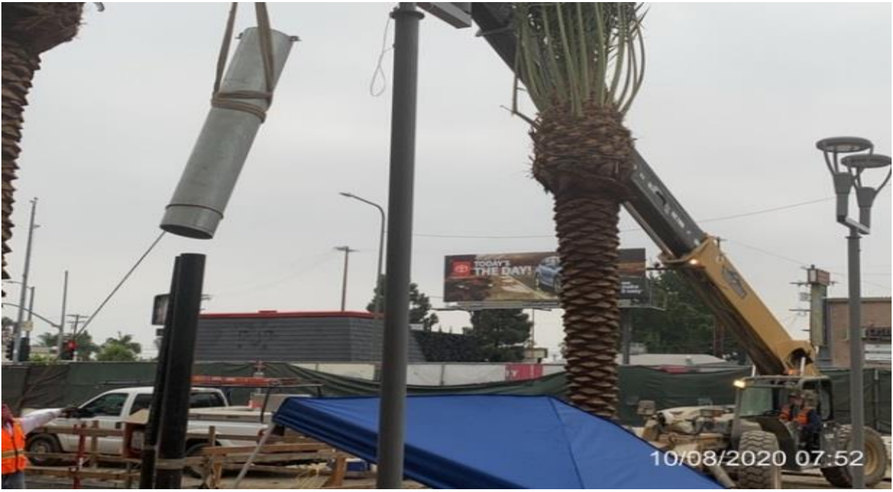
MLK STATION – Installing metal sleeve over the north plumbing vent stack at the plaza level.
