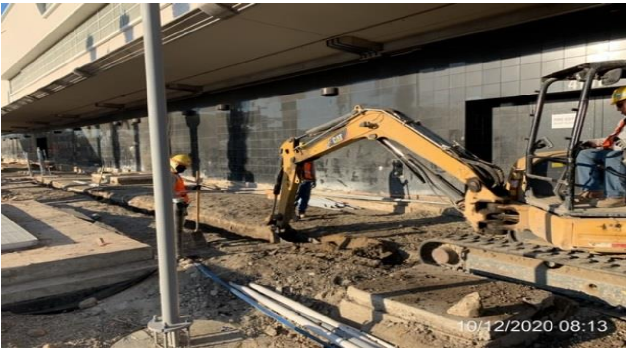
MLK STATION – Continue excavating for CCTV conduit for the pedestrian light poles at the plaza level.
