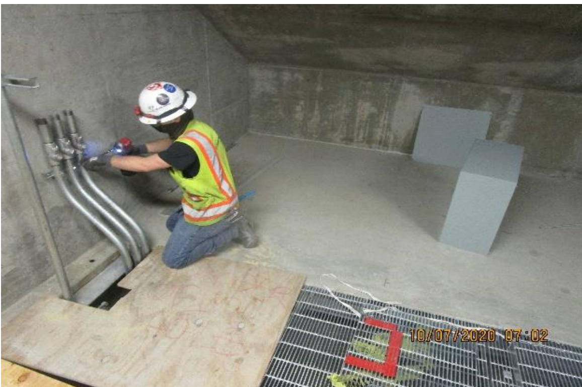
Crenshaw/Vernon – Vernon, Ejector room C134, Continued piping (3) 1-1/4" GRC from SE to 24" PB to SE-6-2X control panel.
