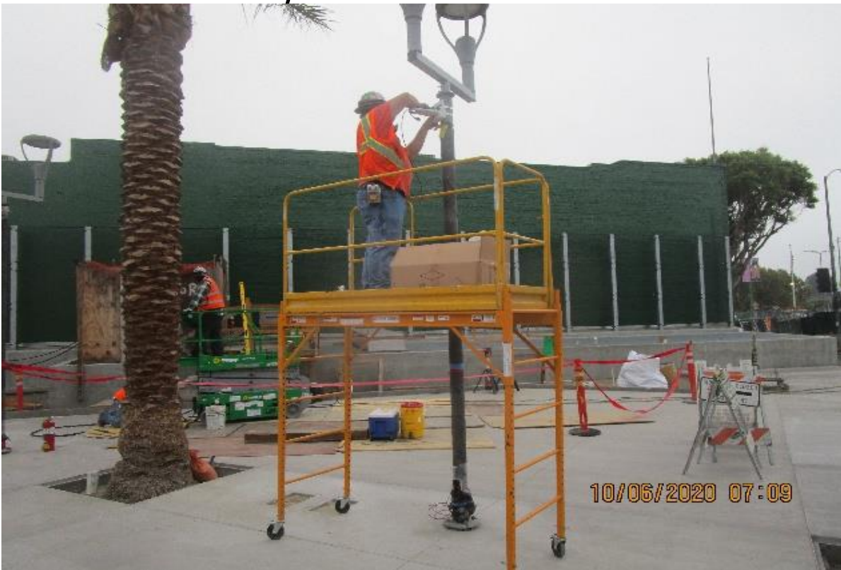
Crenshaw/Vernon – Vernon Plaza, began installing CCTV Camera support brackets at pedestrians' light standard poles.
