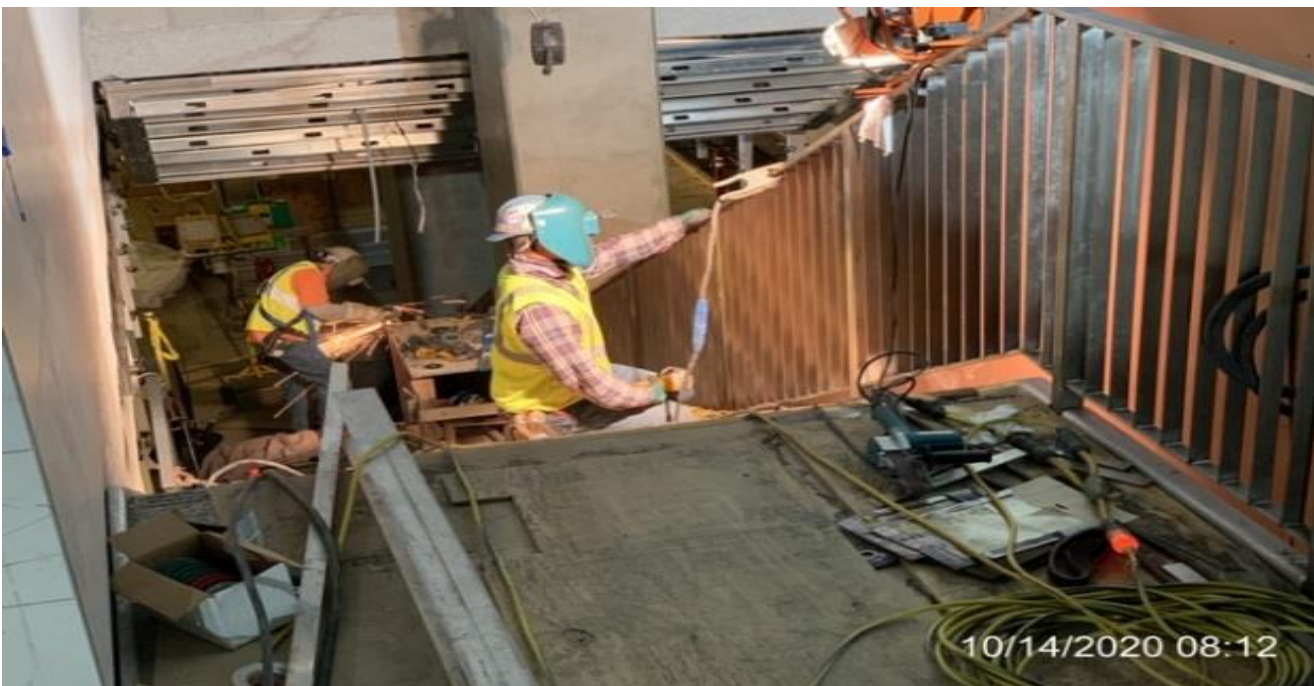
MLK STATION – Continue welding and installing guardrails to Staircase #2 from concourse to platform level.
