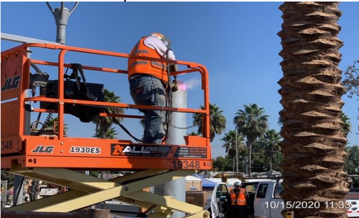
EXPO STATION – WSCC ironworkers welding pipe clamps at top of vent stack.
