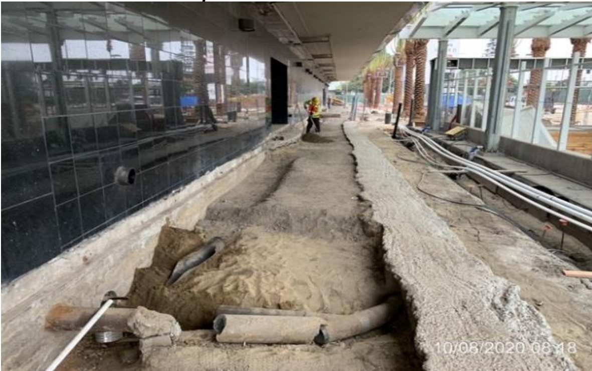
MLK STATION – WSCC crew hand digging to expose damaged drain pipes for repair.
