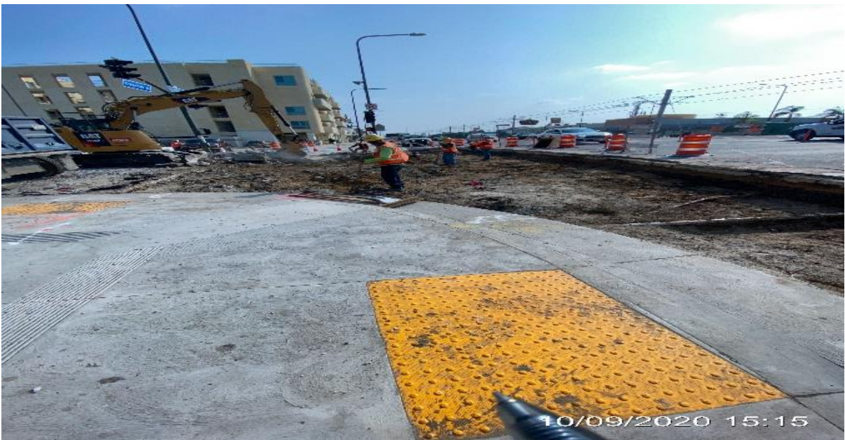
PARK MESA – Excavated/removed 3 concrete road slab sections on the intersection of Crenshaw Blvd and 54th St.
