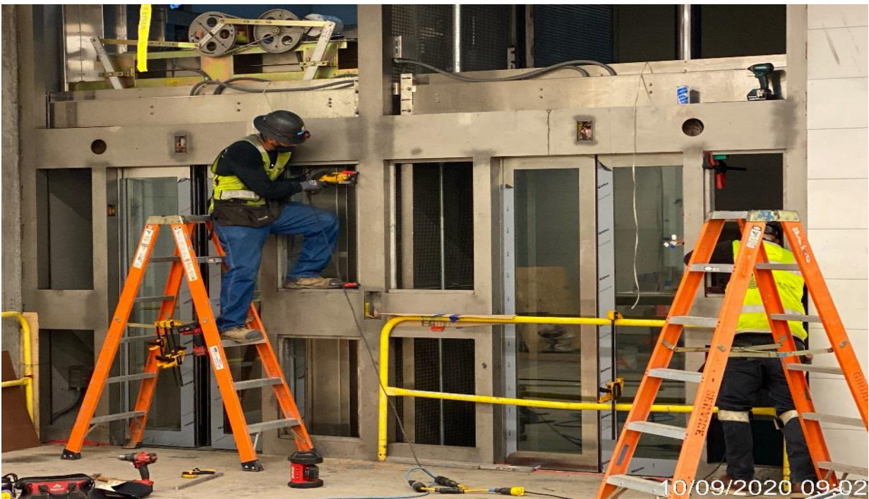
LEIMERT PARK STATION – Installing glass tracks for all 4 Elevators at the concourse level.
