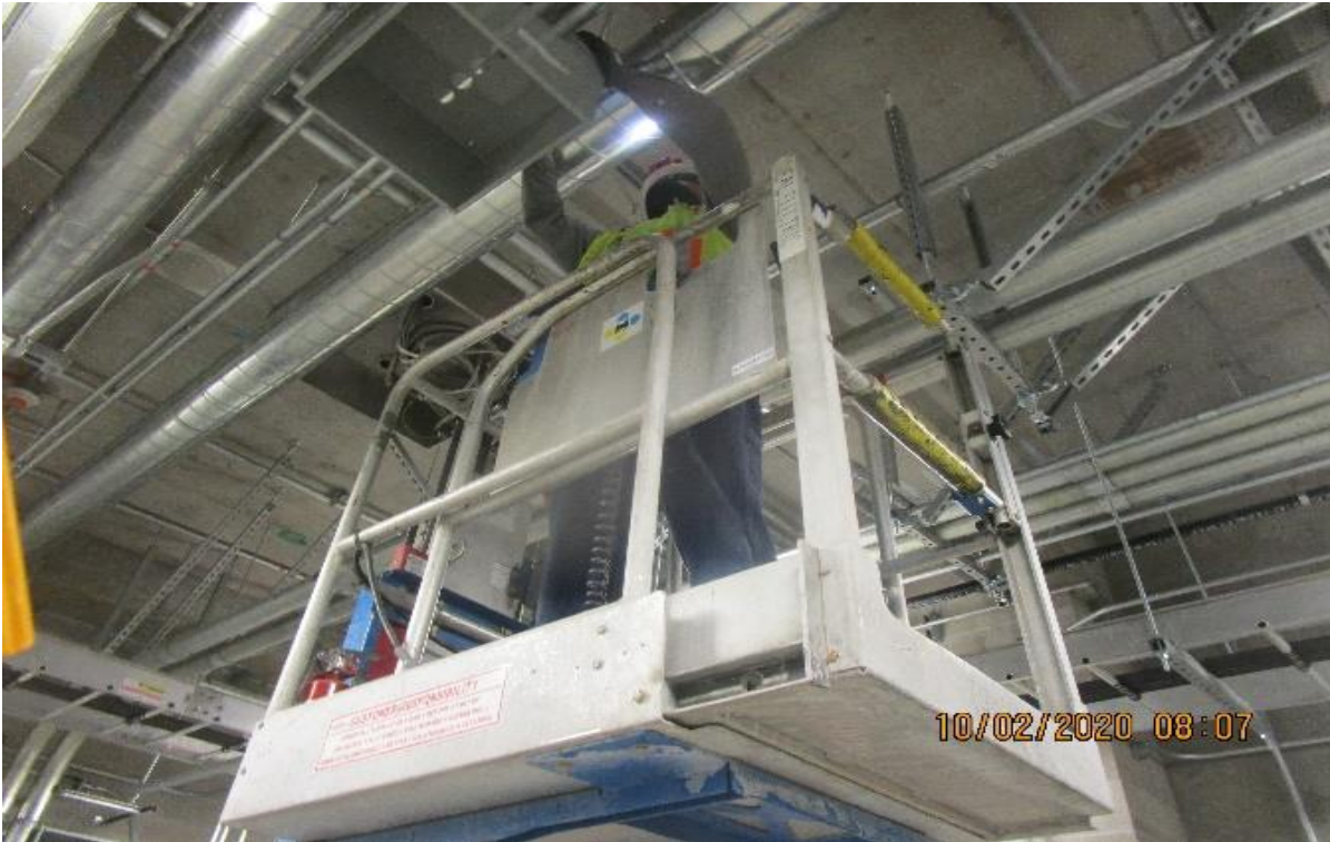
Crenshaw/Vernon – Vernon, Aux power (N) C119 Continued 1-1/4” GRC tie in 18”x18”x12” SCADA PBs MCC2/N to MCC3/N
