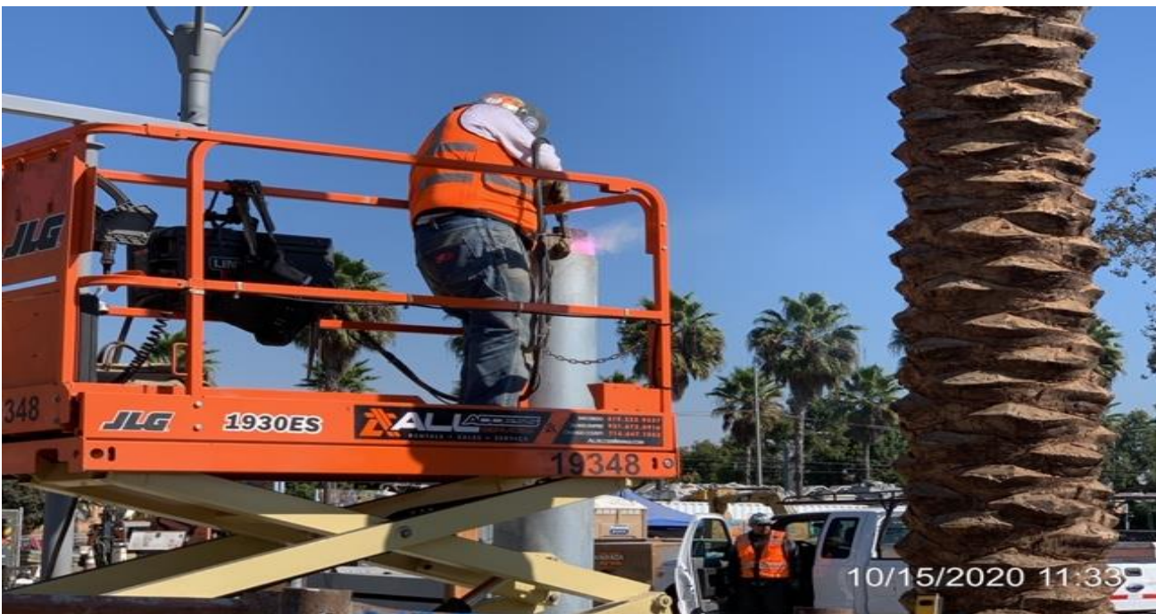
EXPO STATION – Welding pipe clamps to the east plumbing vent stack at the plaza level.
