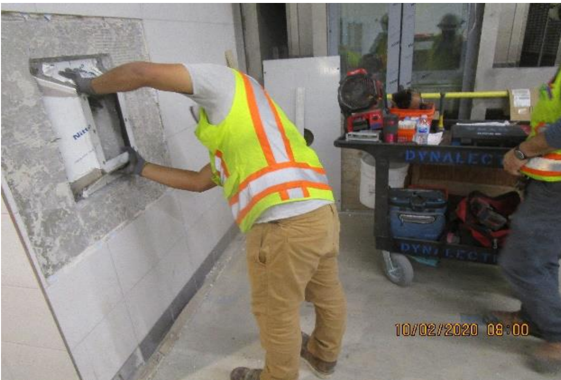
Crenshaw/Vernon – Vernon, Free Area C129, MTEL-17 Resume rework & rough in stainless steel shroud (No Metro Approval)
