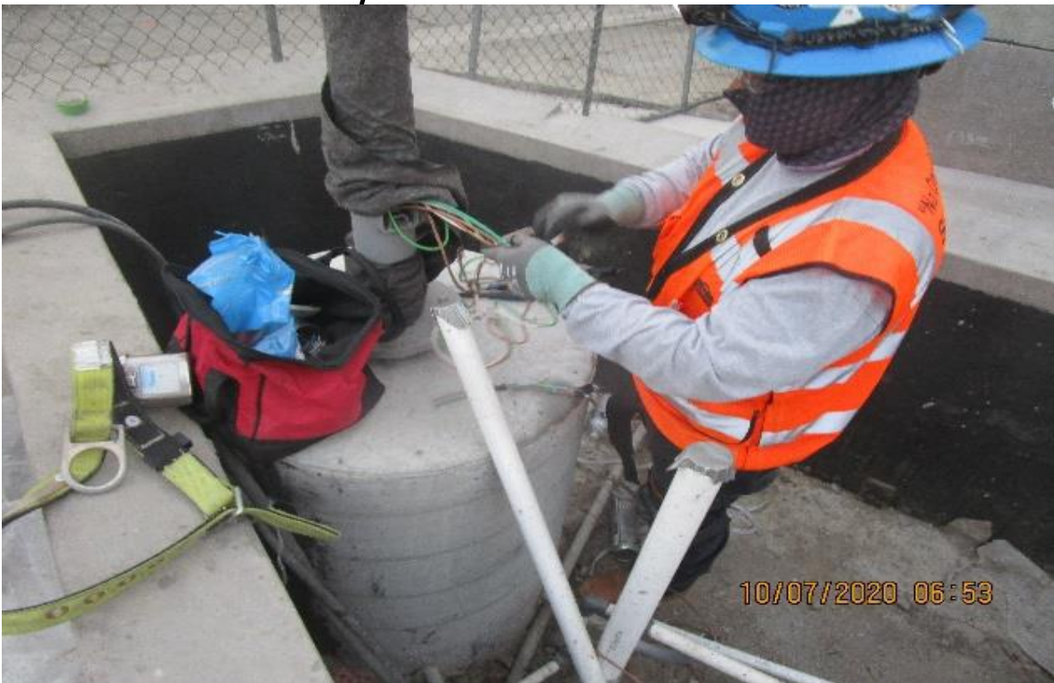
Crenshaw/Vernon – Vernon Plaza, began terminating #10 XHHW-2 load conductors at pedestrian light standard poles.
