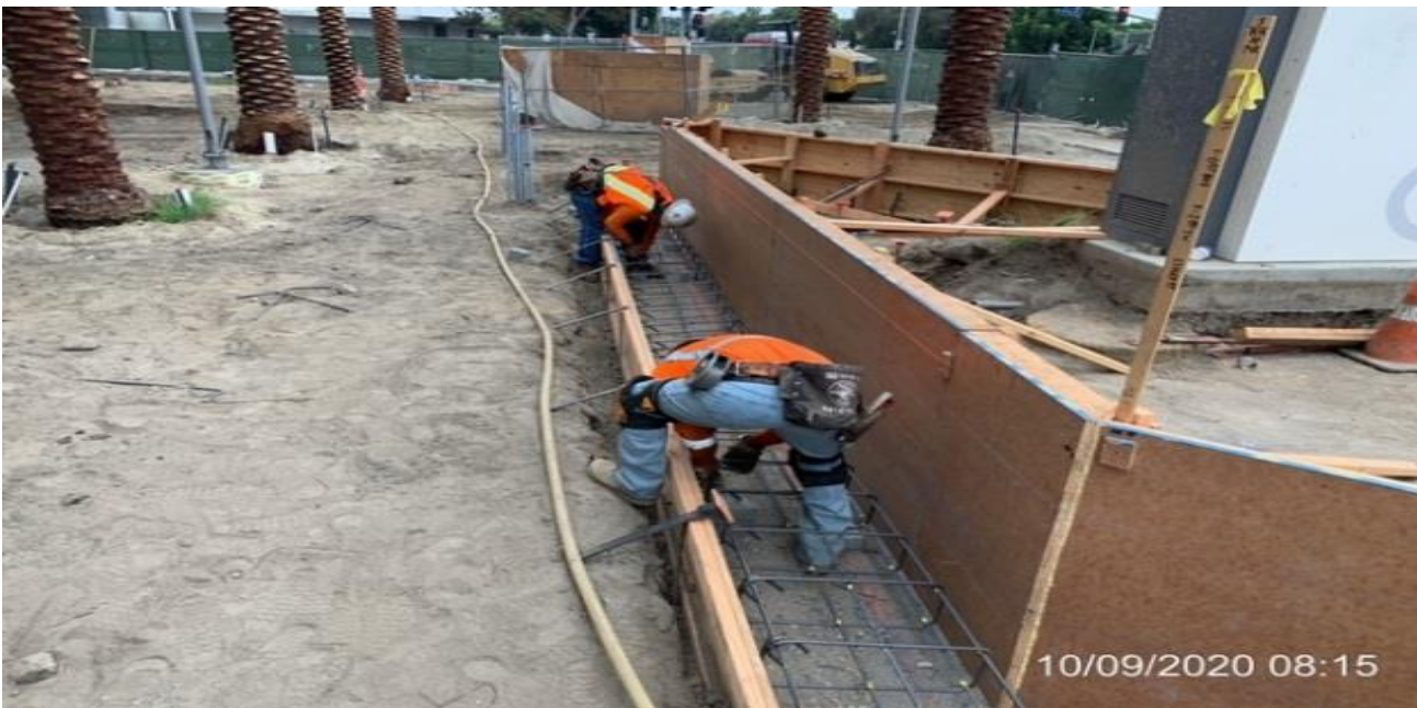
MLK STATION – Installing rebar to the north end planter wall footing at the plaza level.
