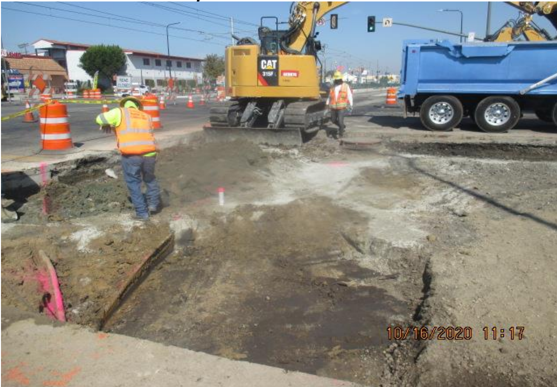
PARK MESA – Excavating/removing road pavement on both north and southbound Crenshaw Blvd and Slauson Ave.
