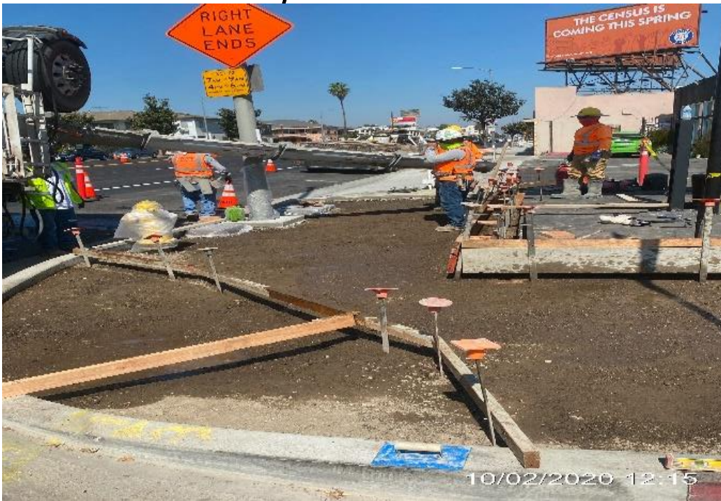
PARK MESA – Placing concrete for new sidewalk and ADA ramp on the northeast corner of 66th St and Crenshaw Blvd.
