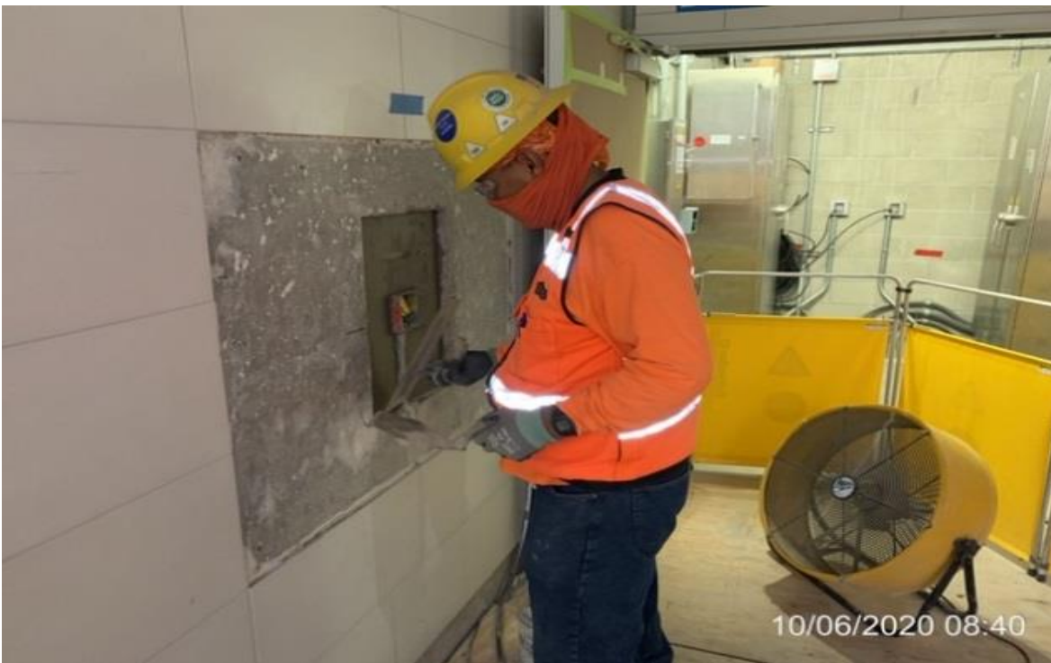
EXPO STATION SITE – WSCC finishers patching and prepping wall for E-tel mount installation.
