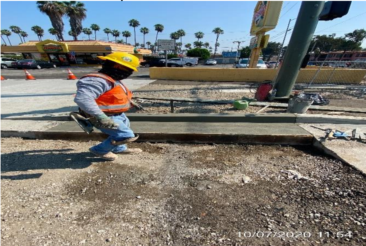
PARK MESA – Placed concrete for new curb/gutter installation on the northeast corner of Crenshaw Blvd and 48th St.
