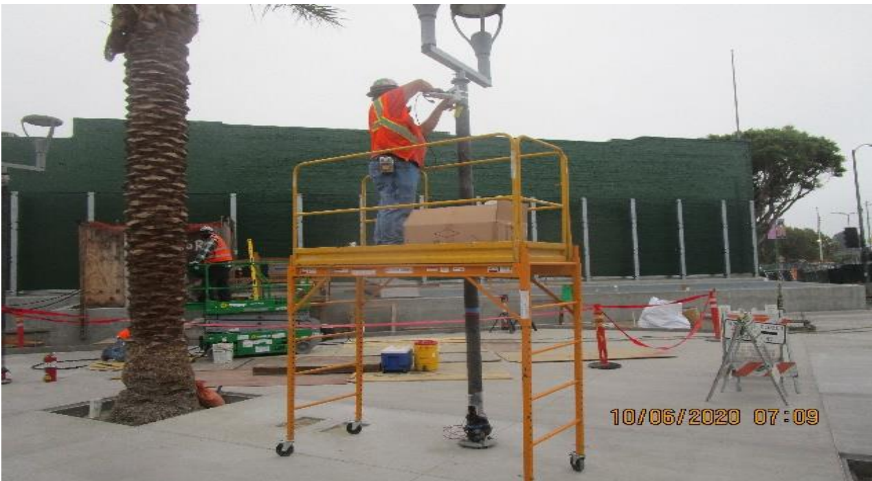
LEIMERT PARK STATION – Installing bracket supports for CCTV installation on the pedestrian light poles at the plaza.
