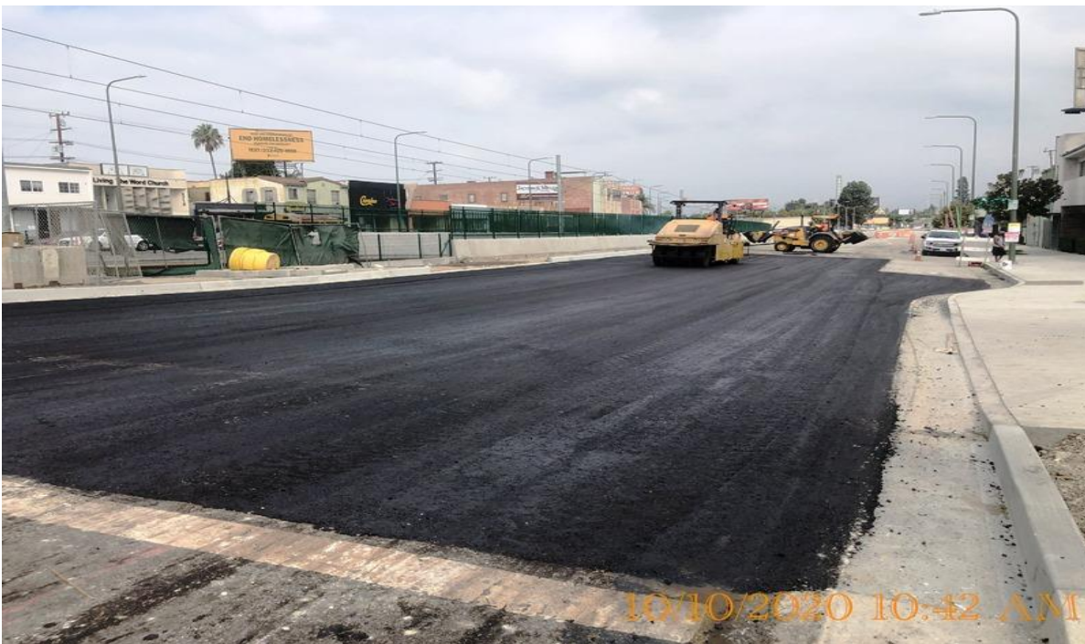
PARK MESA – Placed asphalt concrete and compacted the northbound lanes on Crenshaw Blvd from 48th St to 46th St.
