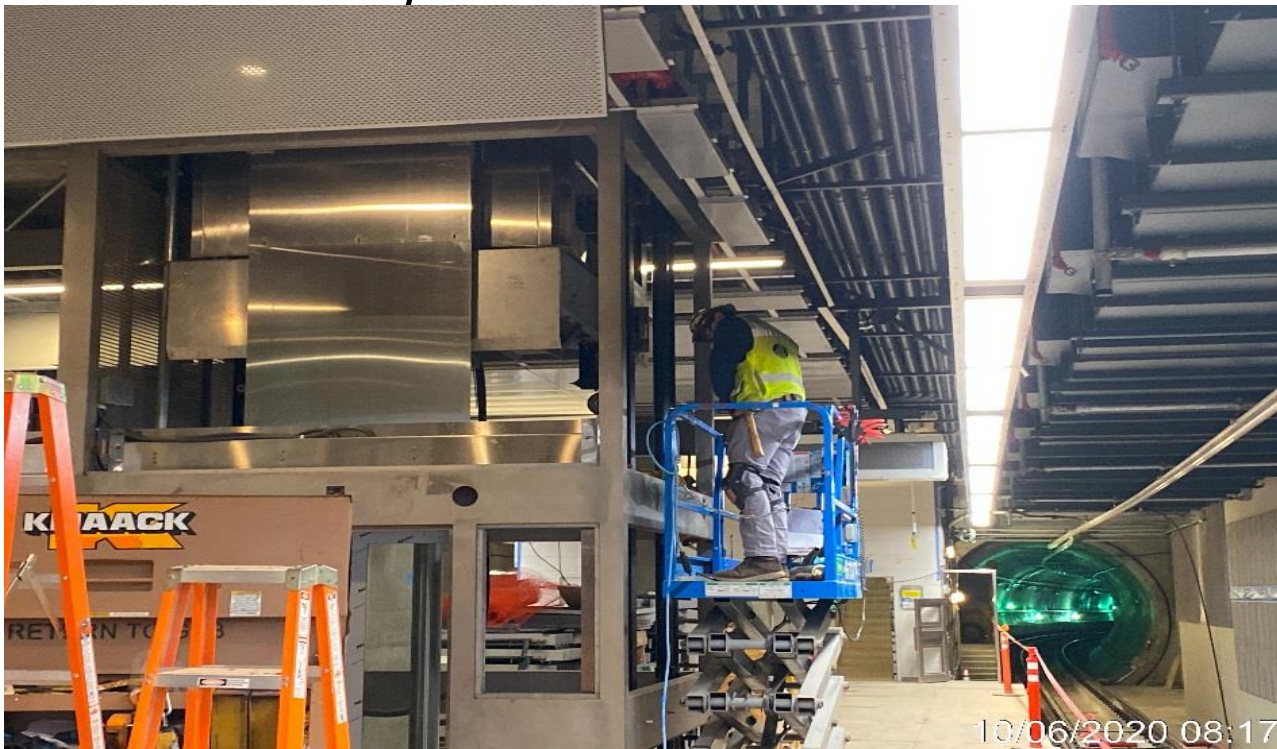
LEIMERT PARK STATION – Continue installing glass tracks for Elevators 3&4 at the platform level.
