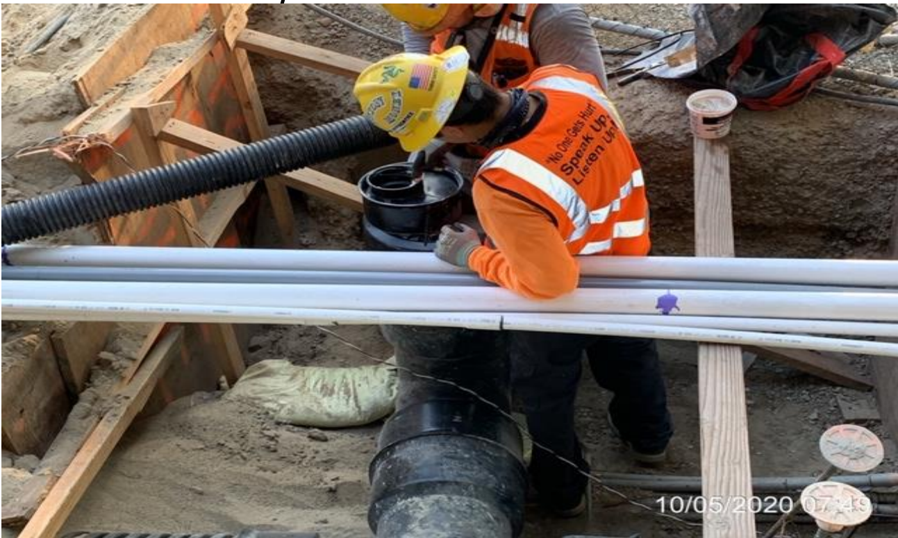
MLK STATION – Installing and connected main entrance canopy gutter drains to the plaza storm drain system.
