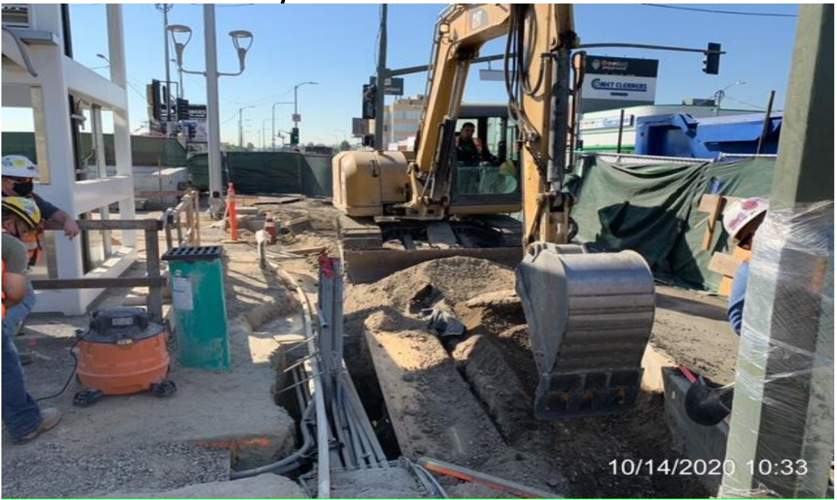
EXPO STATION– WSCC crew trenching for bollards on west side of station.
