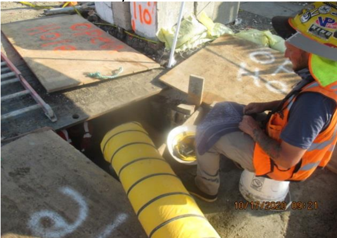
PARK MESA – Sealing interior seams of Storm Drain Line F on northbound Crenshaw Blvd and 60th St.
