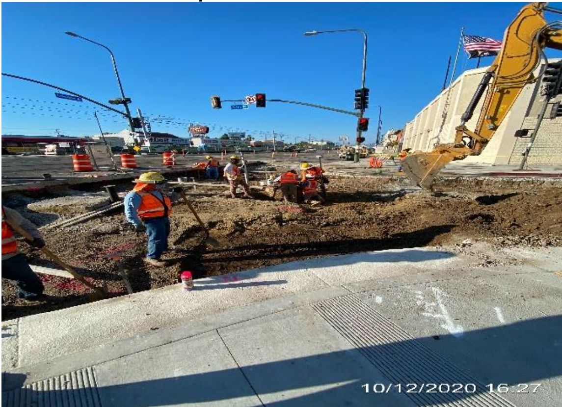
PARK MESA – Excavating north and southbound lanes for restoration on the intersection of Crenshaw Blvd and 57th St.
