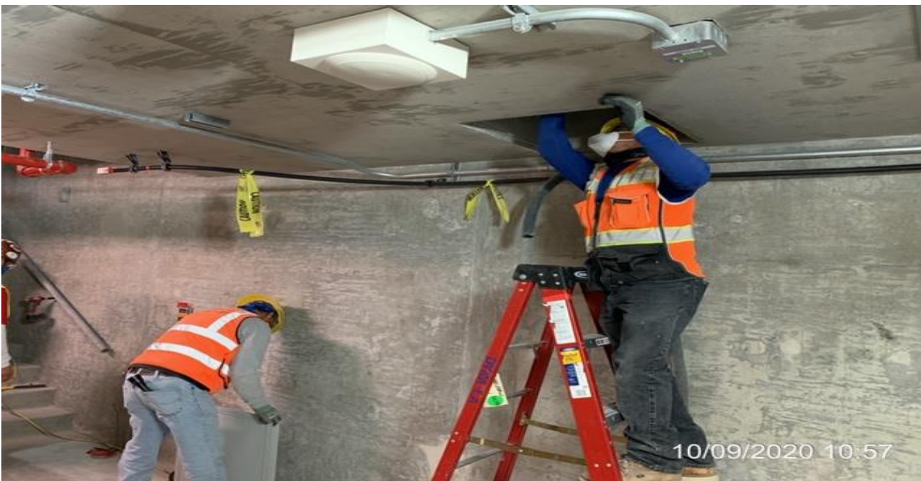
EXPO STATION – Installing ceiling access hatch panels at Emergency Exit Corridors 2&3 at the concourse level.
