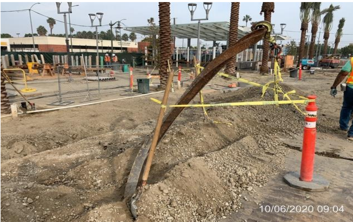
EXPO STATION– Large metal piece observed protruding from yard needs removal.
