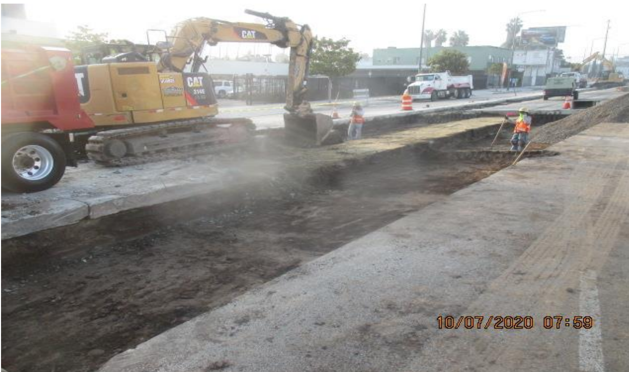
PARK MESA – Backfilling/compacting the northbound lanes and placed rebar on Crenshaw Blvd from 48th St to 46th St.
