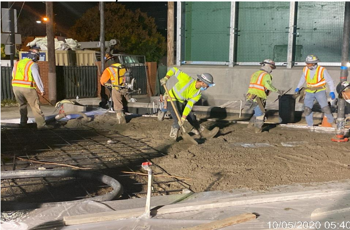
LEIMERT PARK STATION – Continue placing concrete for the architectural topping slab throughout the plaza level.
