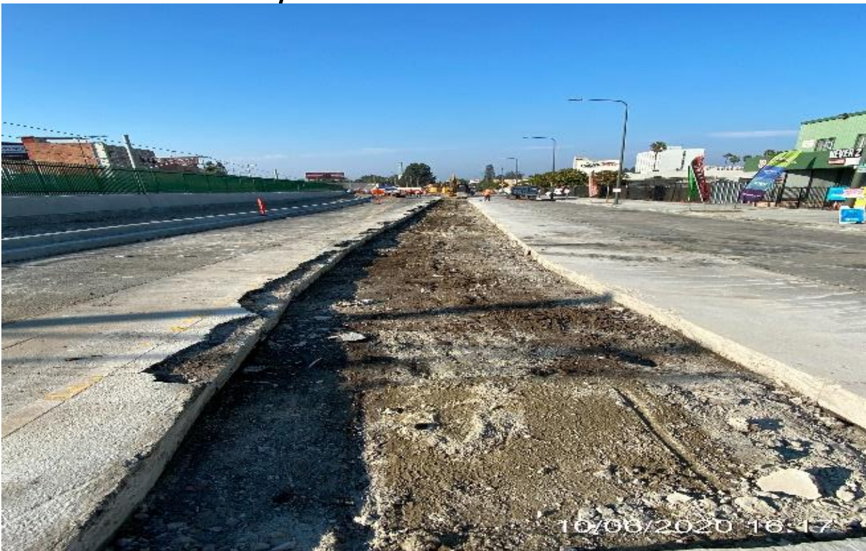
PARK MESA – Excavating northbound lanes for restoration on Crenshaw Blvd from 48th St to 46th St.
