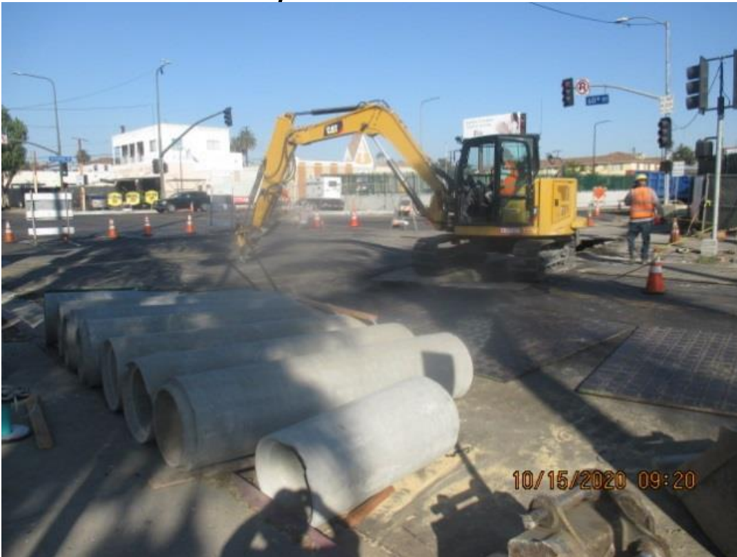
PARK MESA – Continue excavating for Storm Drain Line F on the northeast corner of Crenshaw Blvd and 60th St.
