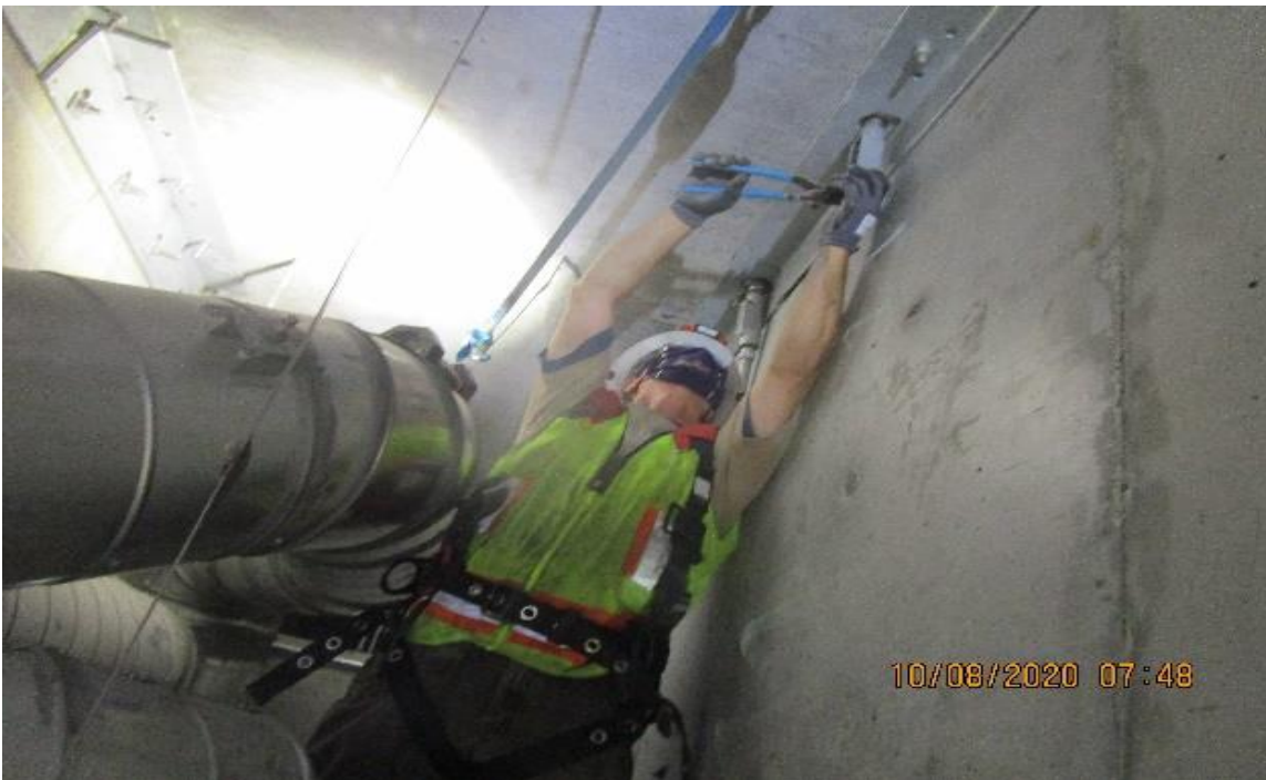
Crenshaw/Vernon – Vernon, above em stair (S) #1 C103 piping 1" GRC & ¾" seal tight conduit to FSD-6-405E & 405F limit switches.
