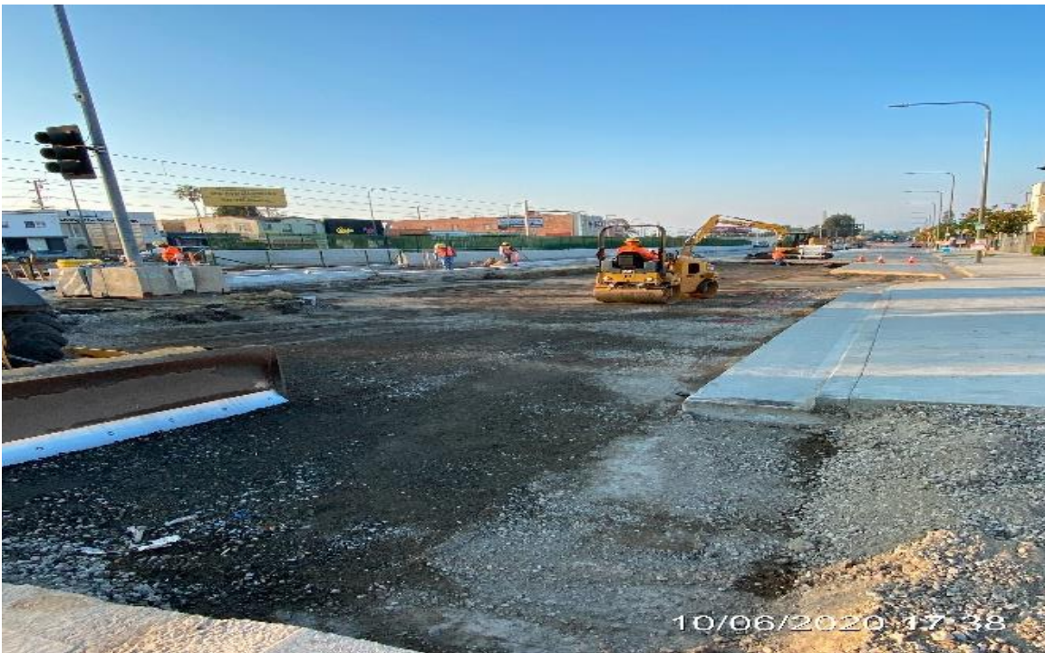
PARK MESA – Continue backfilling and compacting the northbound lanes on Crenshaw Blvd and 48th St.
