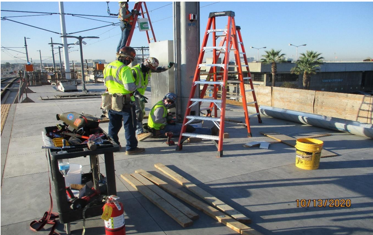
AVIATION/CENTURY- Drilling holes for the stainless steel cladding that mounts on the Aviation Station platform columns
