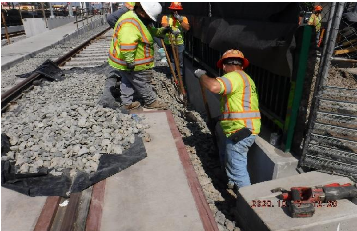
59 th Street – STA 317+70 TK#4/NB looking north – track structure disturbance – 59th St at grade crossing to set conduits for traffic loops .
