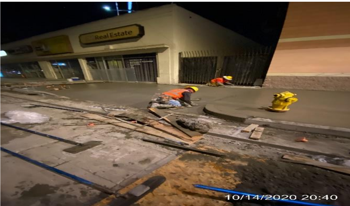
PARK MESA – Continue building formwork and placing concrete for new sidewalk installation along southbound Crenshaw Blvd north of 57th St.
