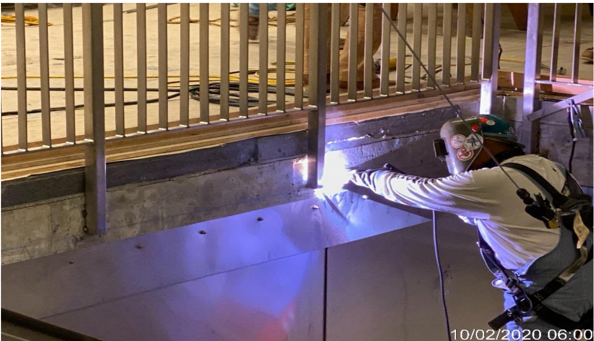
LEIMERT PARK STATION – Continue welding guardrails around the opening entrance of Staircase #4 and Escalator #6 at the concourse.
