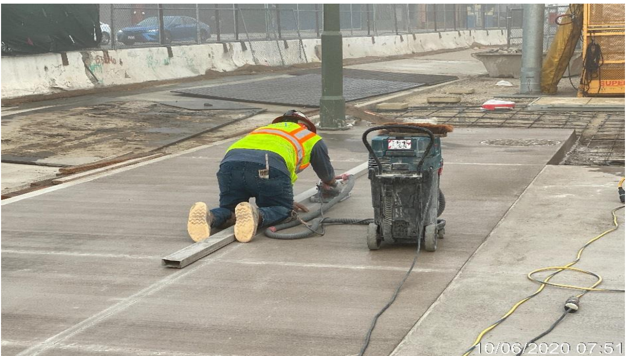
LEIMERT PARK STATION – Continue saw cutting control joints for the architectural topping slab throughout the plaza level.
