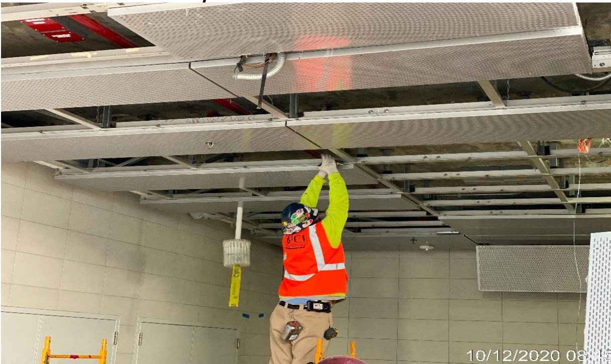
LEIMERT PARK STATION – Resume ceiling panel installation throughout the Free & Paid Area of the concourse level.
