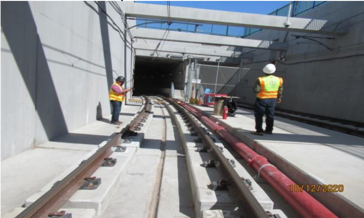
UG1- Field walk with Metro CM team at UG1 south portal SB track STA 281+90 to evaluate cut & cover wall (looking north)
