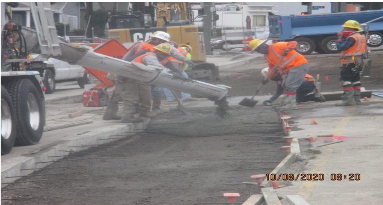
PARK MESA – Placing concrete for the northbound lanes on Crenshaw Blvd from 48th St to 46th St.
