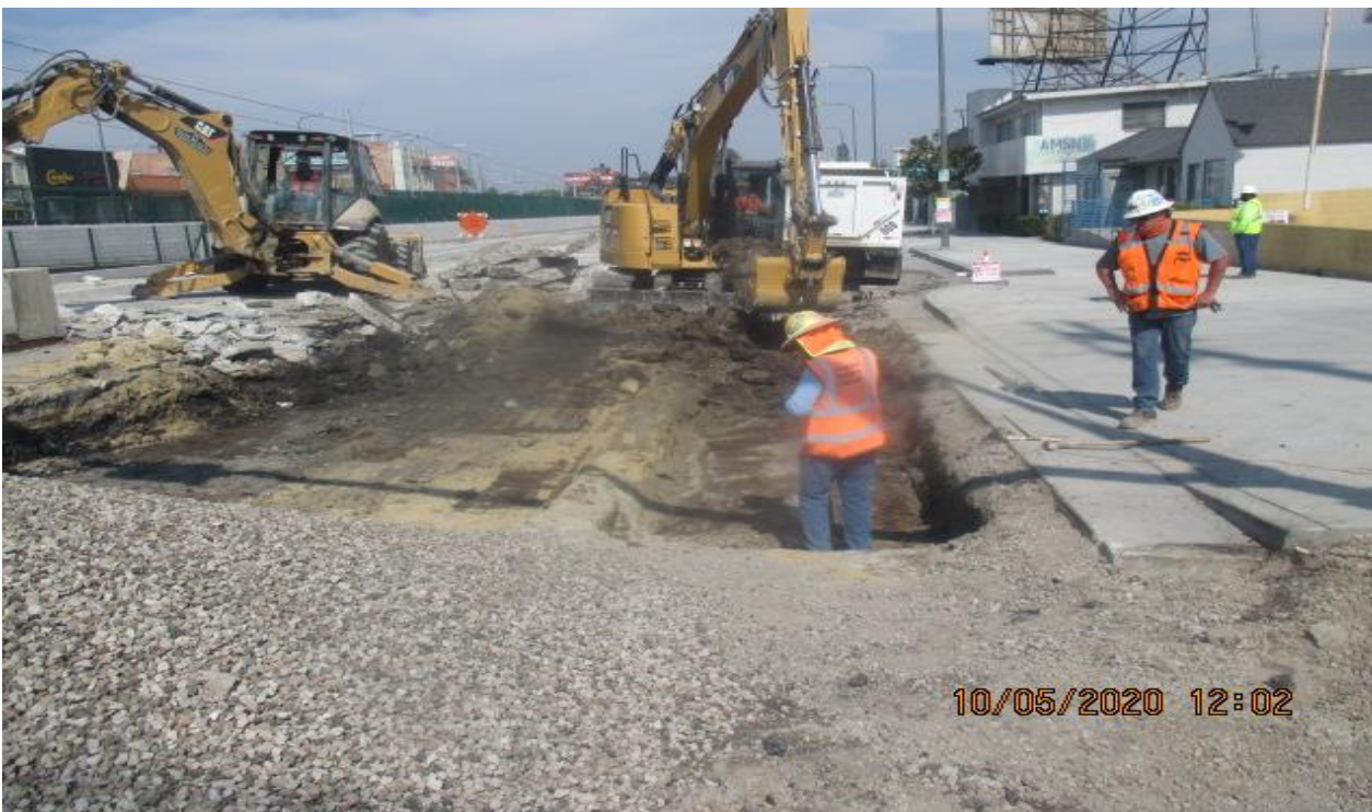
PARK MESA – Excavating northbound lanes for restoration on Crenshaw Blvd and 48th St.
