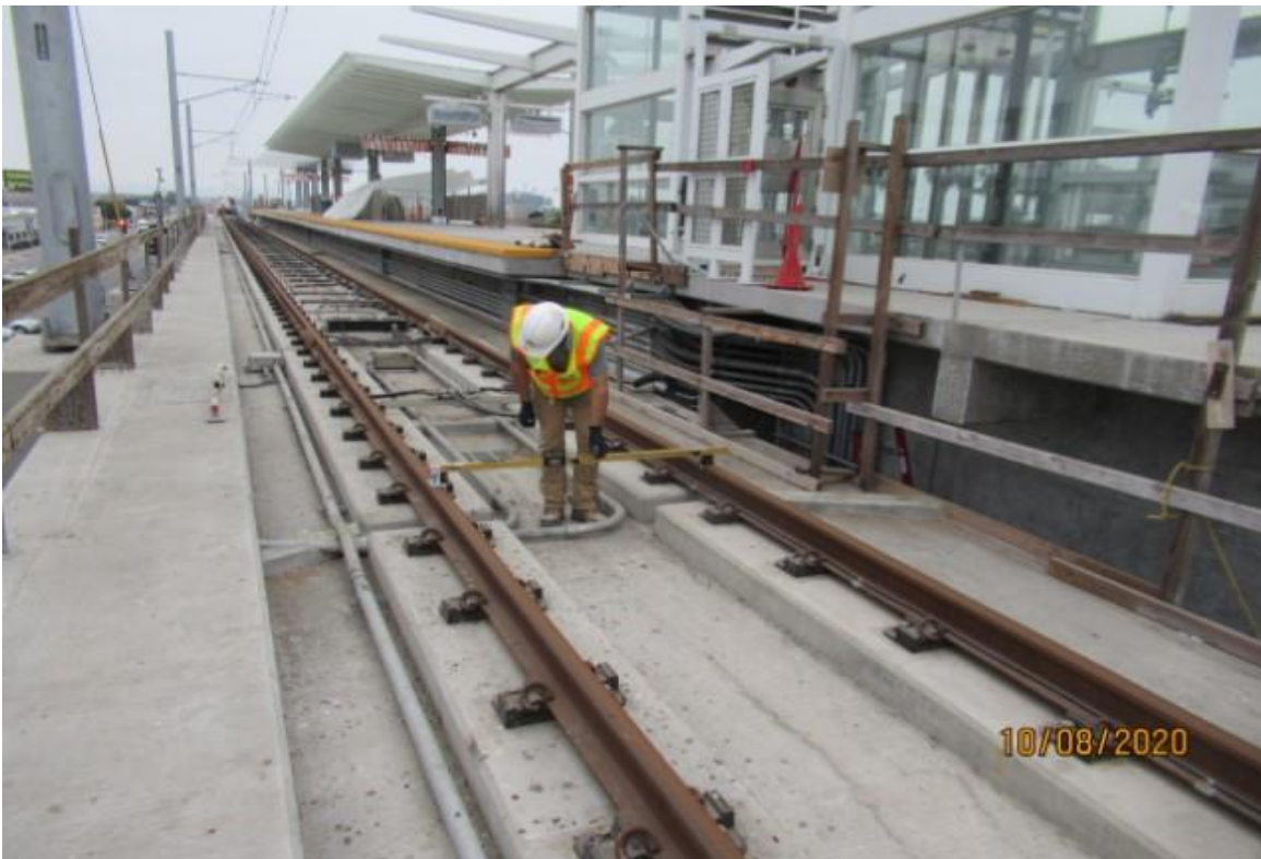
AVIATION/CENTURY- Metro QA track inspector verifying track cross level & gauge on SB track on Century/Aviation OP. Part of field walk (looking northeast)
