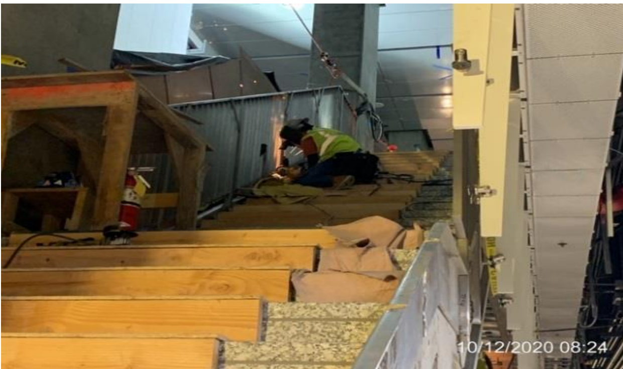
MLK STATION – Continue welding and installing guardrails to Staircase #2 from concourse to platform level.
