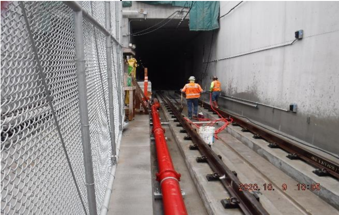
UG3 – STA 311+35 TK#3/SB looking south – invert cleaning UG3 in progress (north portal).
