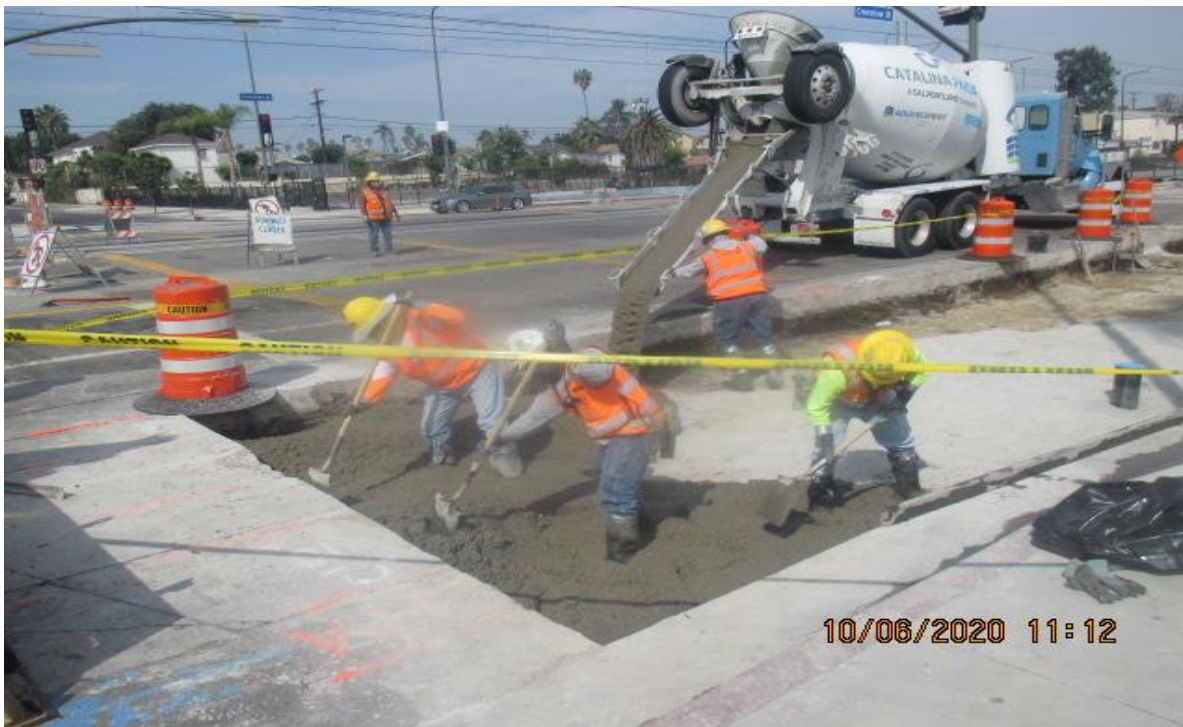
PARK MESA – Placing slurry backfill and concrete over the northbound lanes on Crenshaw Blvd and 52nd St.
