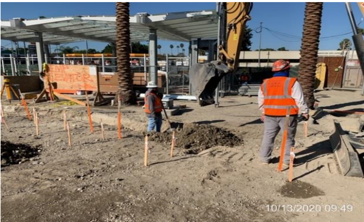
EXPO STATION – WSCC crew trenching for bollards on east side of station.
