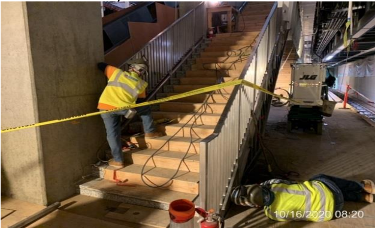
MLK STATION – Continue welding and installing guardrails to Staircase #2 from concourse to platform level.
