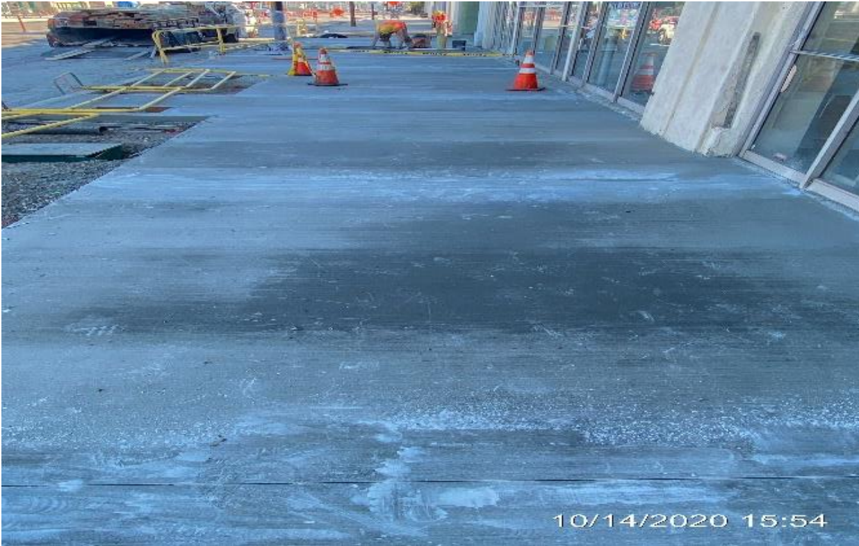
PARK MESA – Saw cut new sidewalk panels on southbound Crenshaw Blvd and 57th St.
