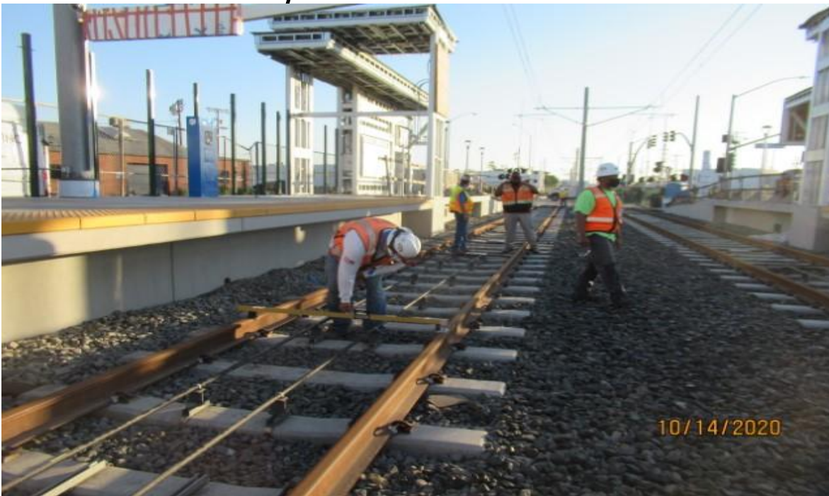
Hindry – Field walk with WSCC & Metro CM personal at Hindry station, evaluating track & overall guideway condition (looking north)
