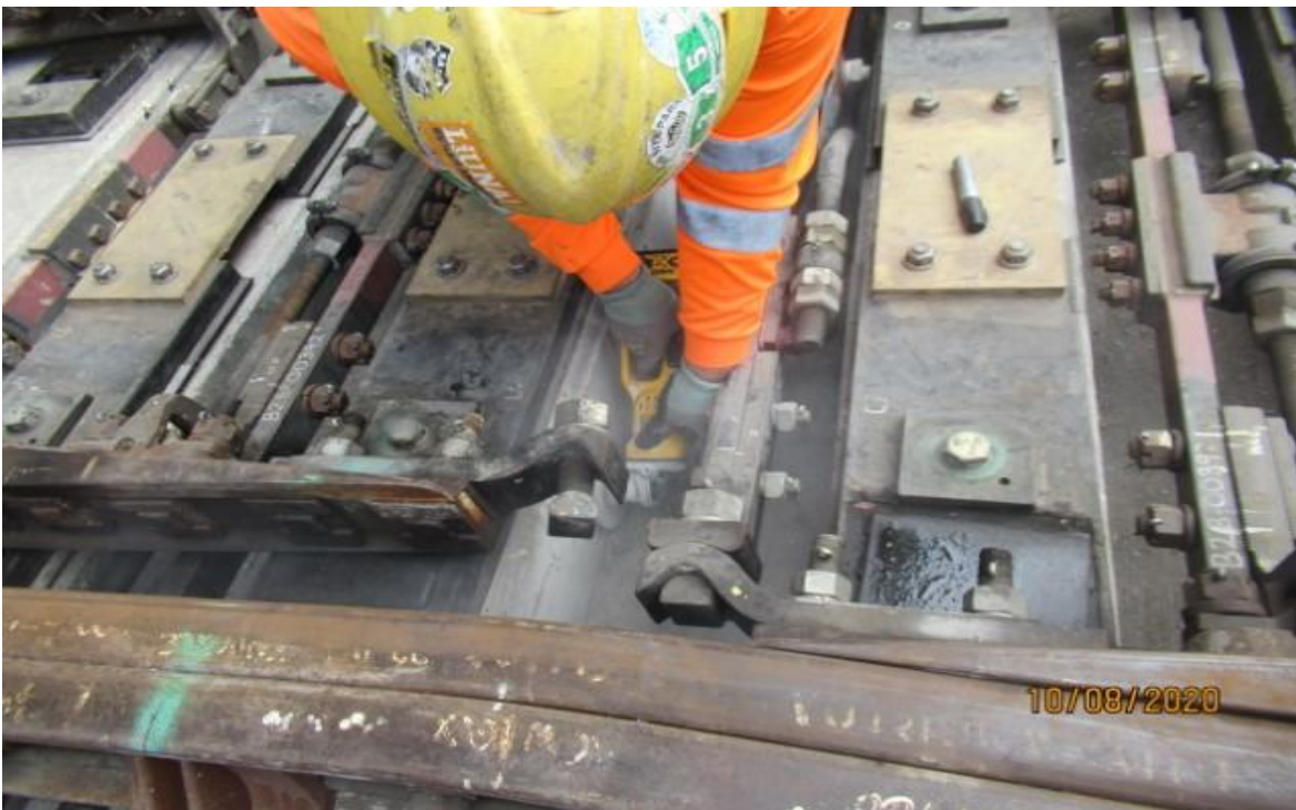
Guideway- WSCC using hand grinder to shave down switch machine plinth, to clear point protector rod at GL Wye Rework
