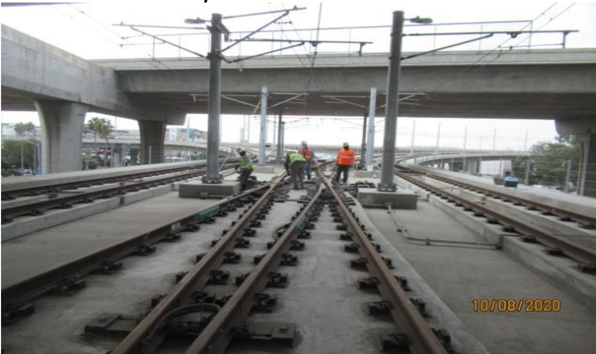
Guideway- WSCC/LKC personal at GL Wye for MPF repair work on plinth (looking south) Rework
