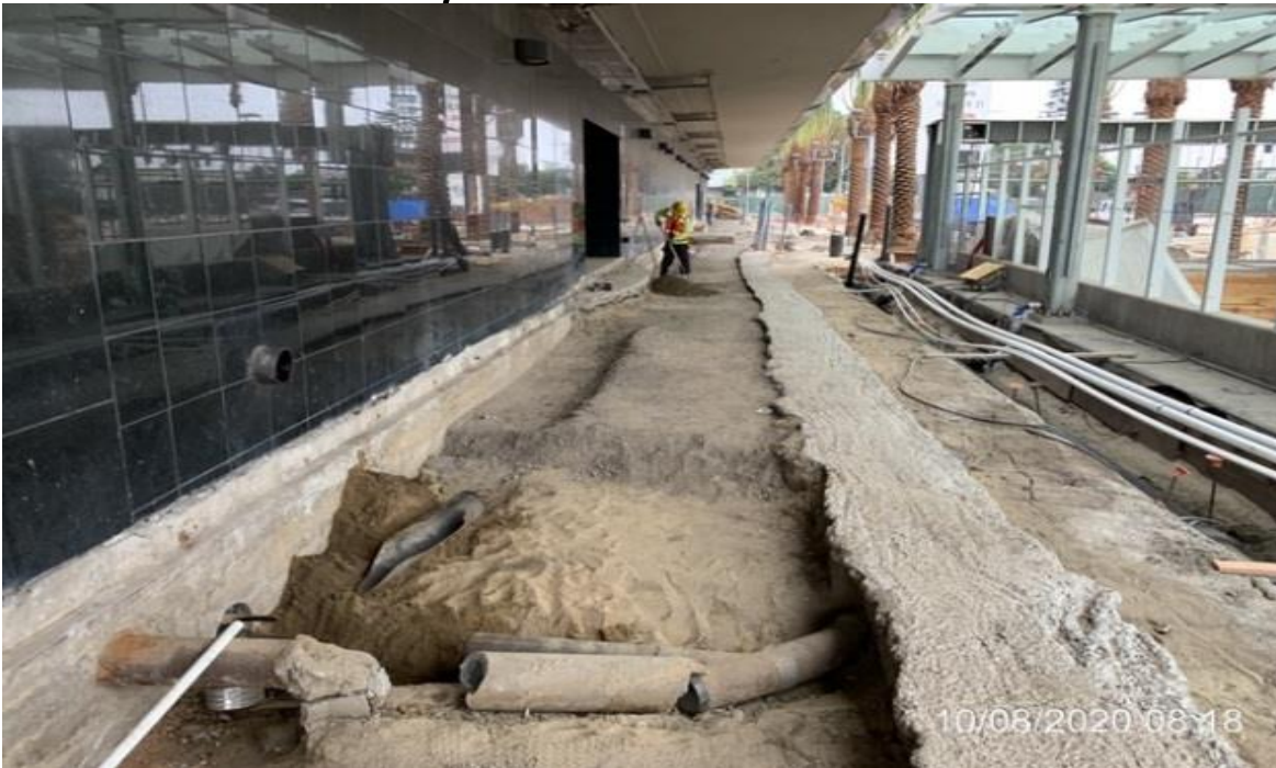
EXPO STATION SITE – WSCC crew hand digging to expose damaged drain pipes for repair.
