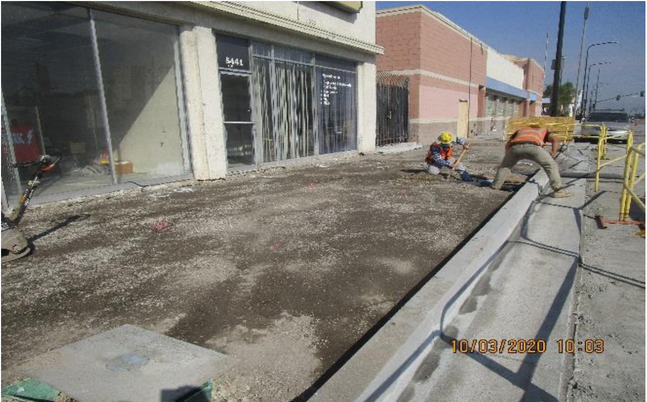
PARK MESA – Installed drains at the curb and gutter along SB Crenshaw Blvd between 54th and 57th St.
