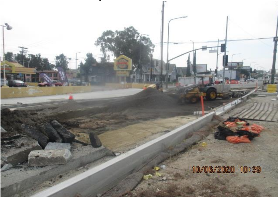
PARK MESA – Continue excavating northbound lanes and backfilled on Crenshaw Blvd and 48th St.
