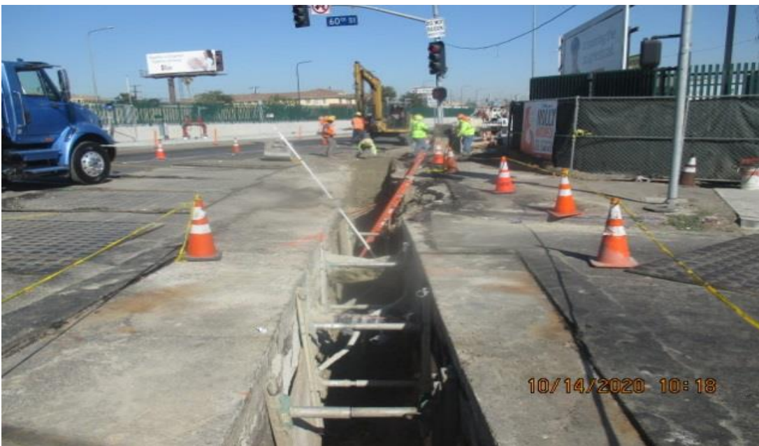
PARK MESA – Continue excavating for Storm Drain Line F on the northeast corner of Crenshaw Blvd and 60th St.
