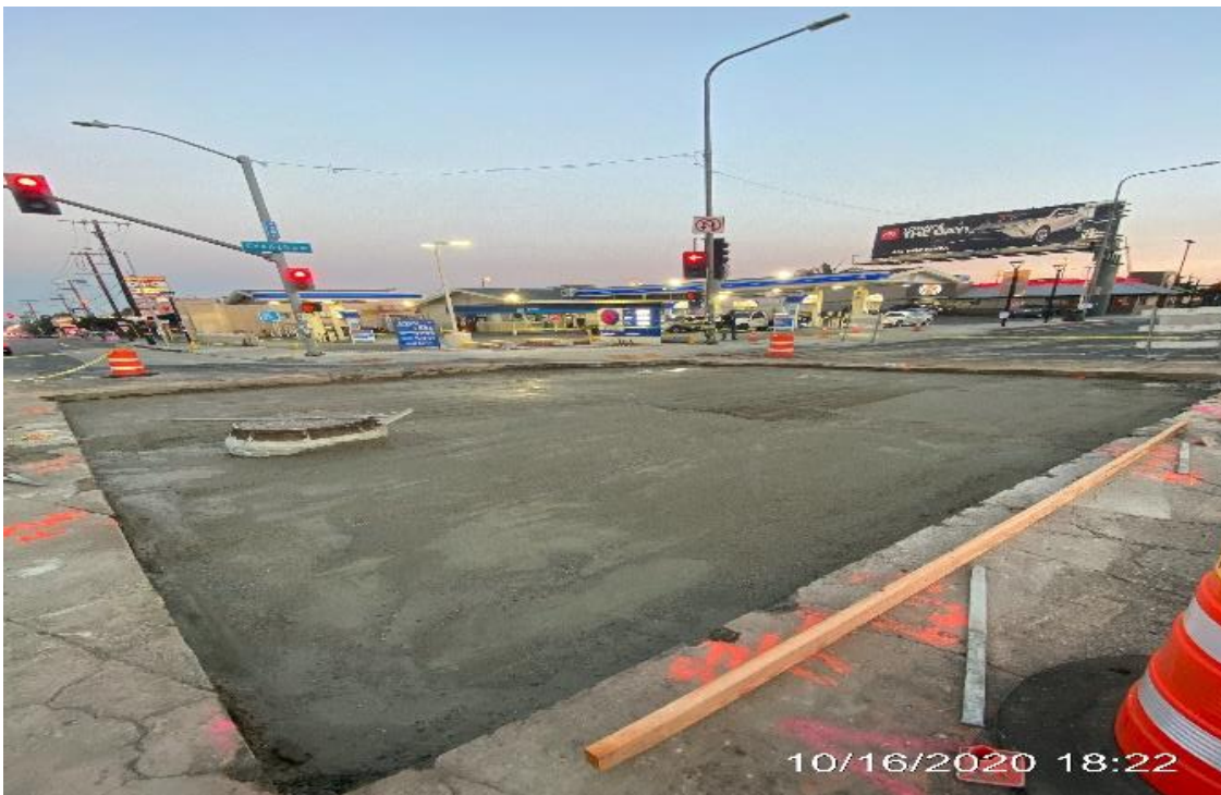
PARK MESA – Built formwork, placed rebar and concrete over north and southbound lanes on Crenshaw Blvd and Slauson Ave.
