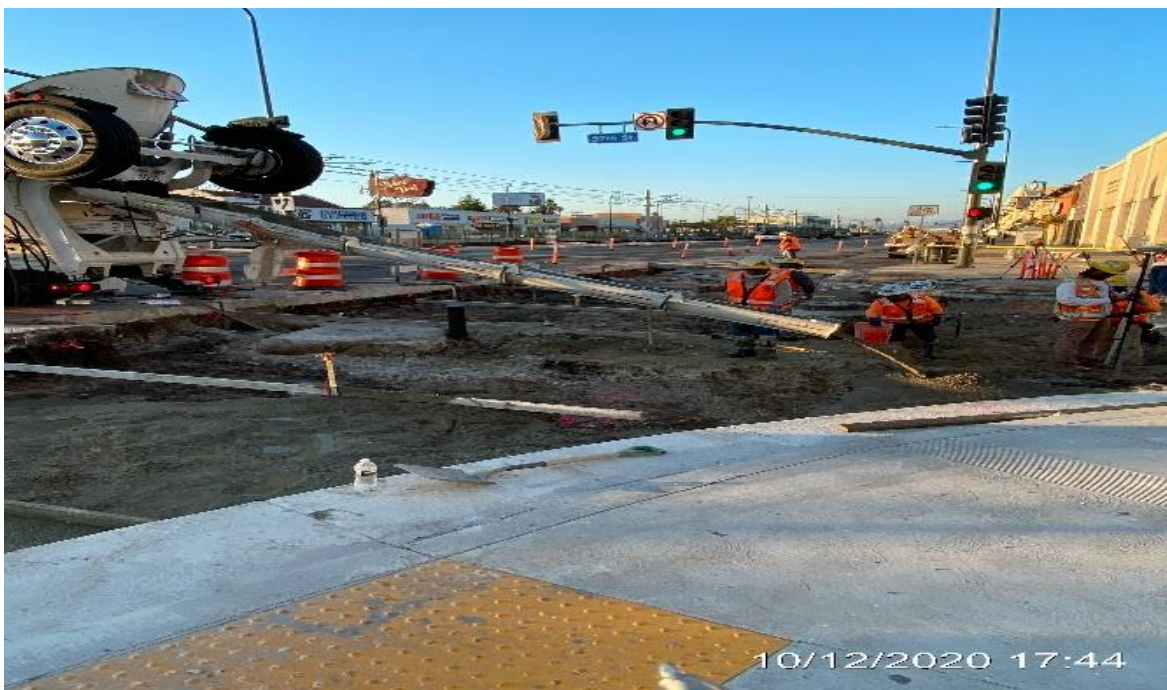
PARK MESA – Building formwork and placing concrete on the north and southbound lanes for restoration at the intersection of Crenshaw Blvd and 57th St.
