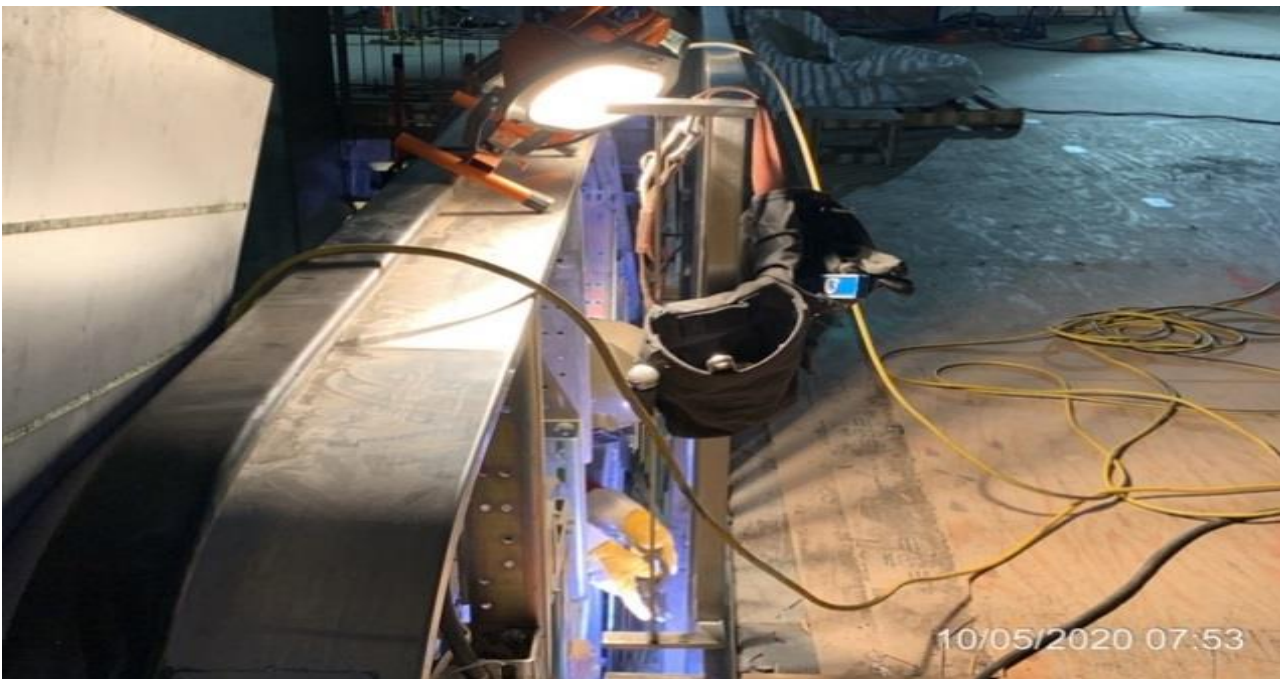
MLK STATION – Continue welding and finalizing guardrail finishes for Staircase #3 from concourse to platform level.
