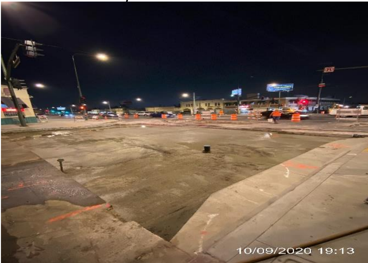
PARK MESA – Placed forms and slurry for 3 sections on the intersection of Crenshaw Blvd and 54th St.
