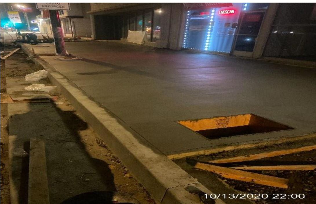
PARK MESA – Build formwork and placed concrete for new sidewalk installation on southbound Crenshaw Blvd and 57th St.
