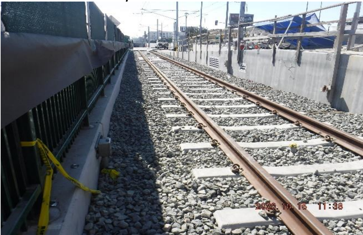
59 th Street – STA 319+16 TK#4/NB looking south – north limit of current track structure disturbance (backfilled) – 59th St at grade crossing to set conduits for traffic loops Slauson.
