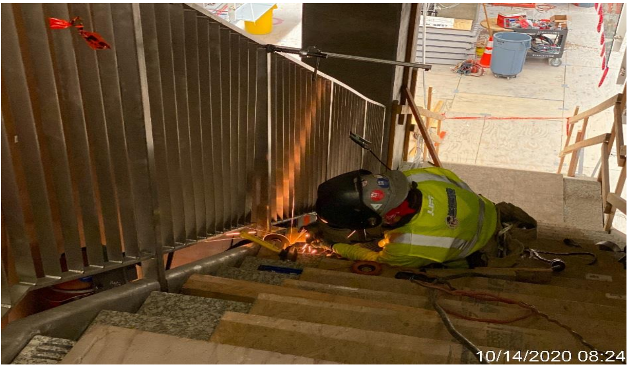
LEIMERT PARK STATION – Continue welding guardrails for Staircases 3&4 from concourse to platform level.
