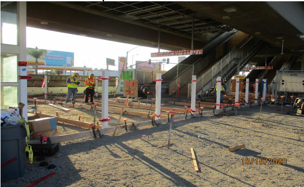
AVIATION/CENTURY- Fire alarm strobe light installation at the Aviation Station ticket kiosk.
