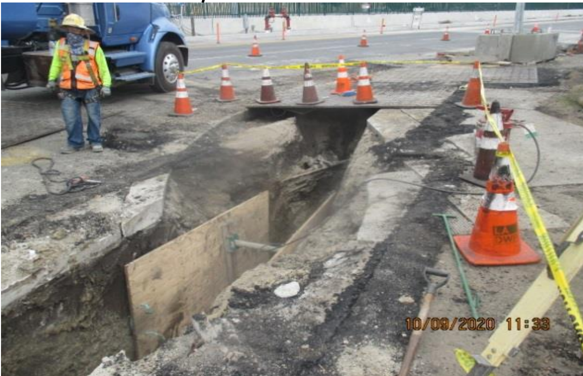
PARK MESA – Continue excavating for Storm Drain Line F on the northeast corner of Crenshaw Blvd and 60th St.
