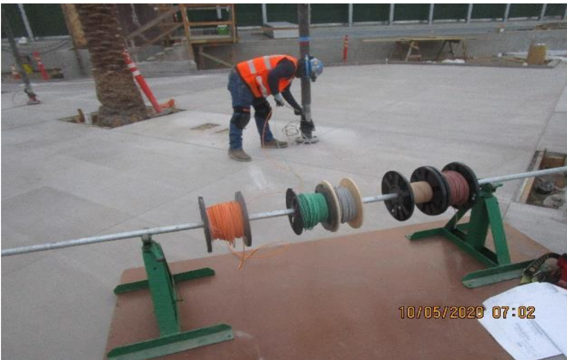
Crenshaw/Vernon – Vernon Plaza, continued pulling (3) #10 XHHW-2 wiring to Pedestrian light standards from embedded PB's.
