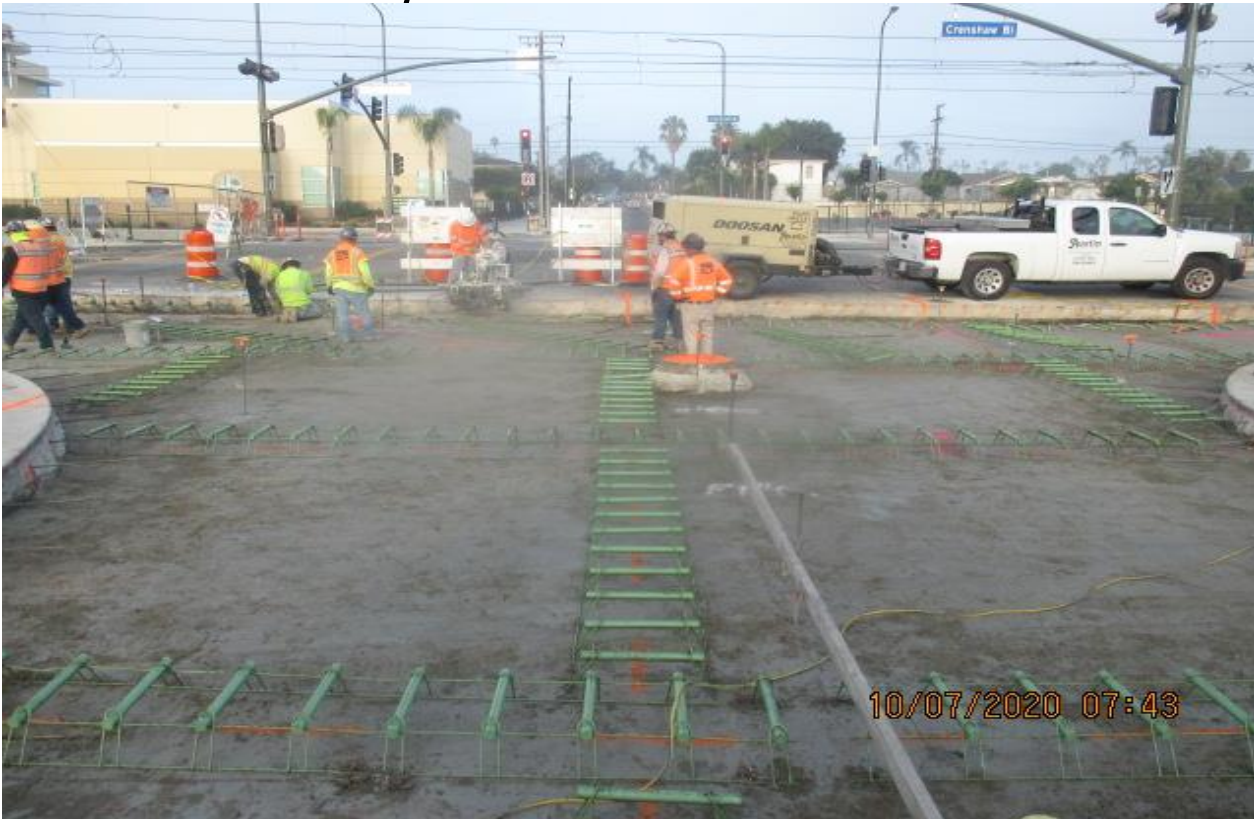
PARK MESA – Placing rebar in preparation for concrete placement of the existing roadway slab on Crenshaw Blvd and 52nd St.
