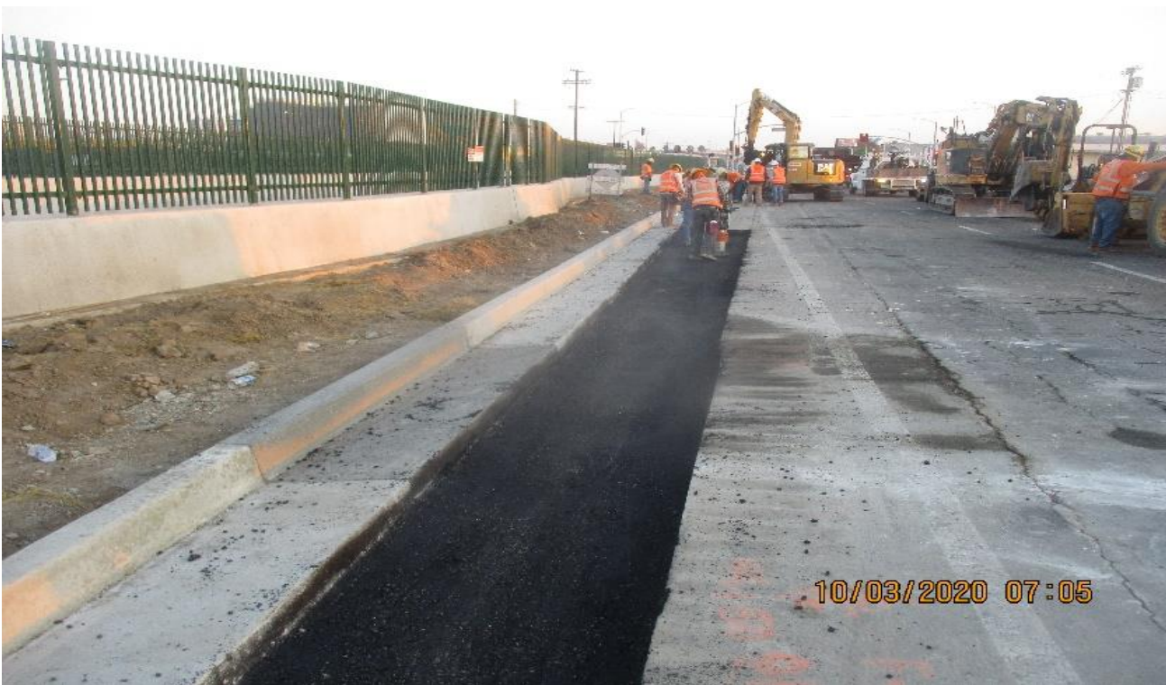
AVIATION/CENTURY- WSCC Slot paved along gutter out 104th to S/end of UG-1 on S/B Aviation.
