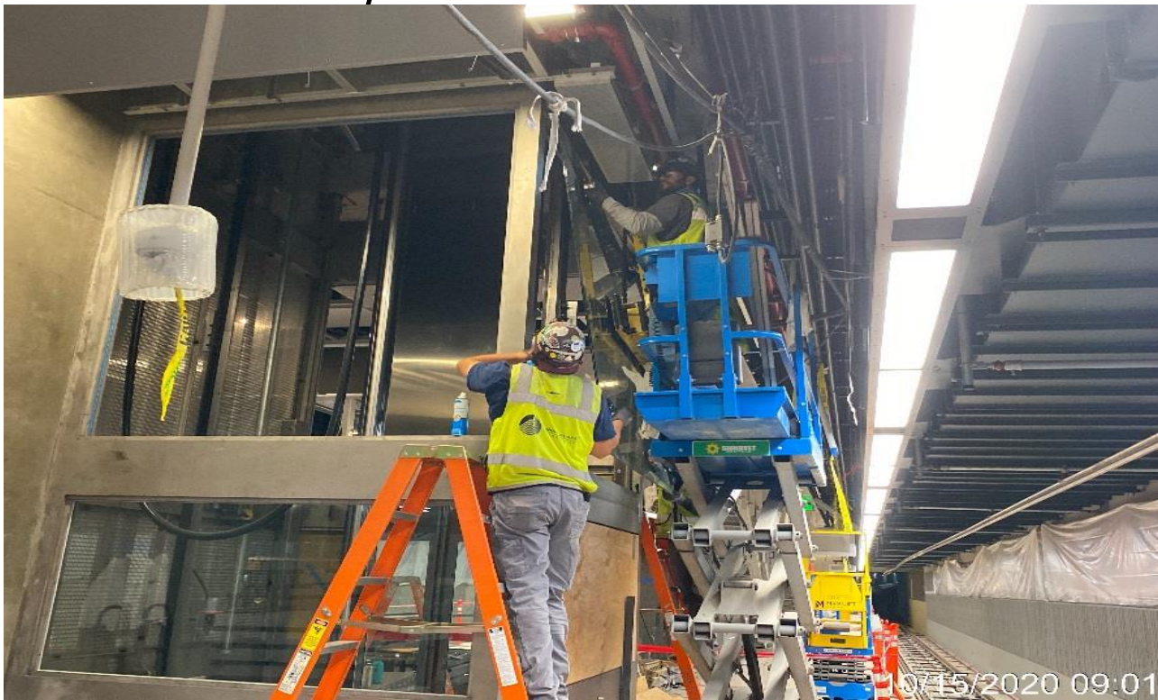
LEIMERT PARK STATION – Continue installing glass tracks for Elevators 3&4 at the platform level.
