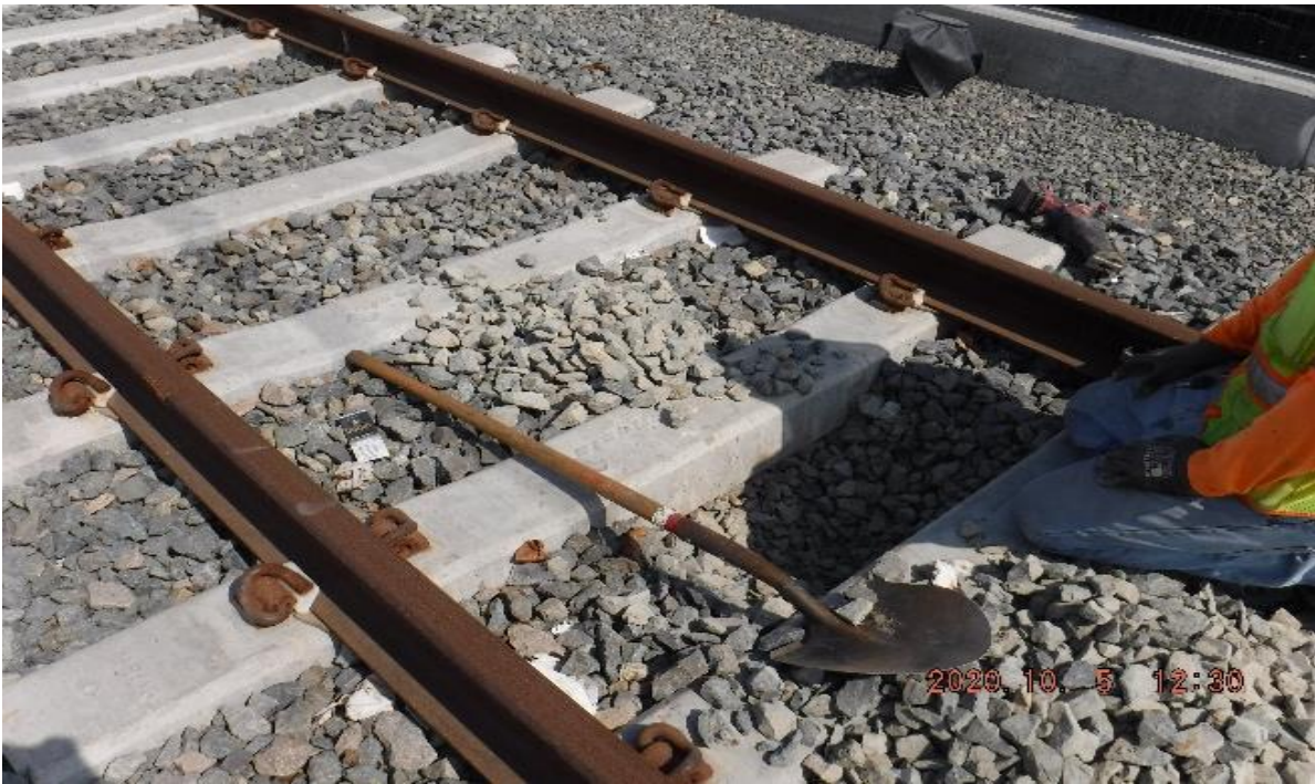
57 th Street – STA 331+15 TK#4/NB looking north – track ballast disturbance in search for traffic loops conduits north of 57th at grade crossing – PUNCH LIST
