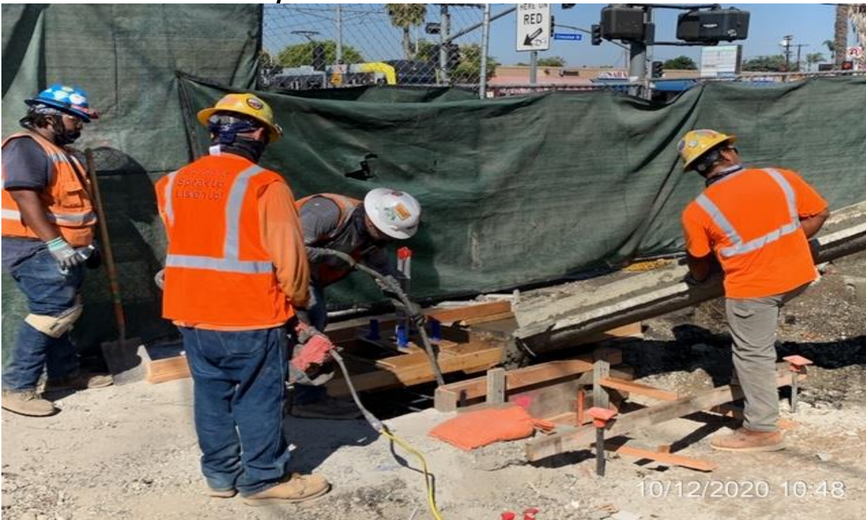
EXPO STATION – Placing concrete for the grand pylon foundation footing at the plaza level.
