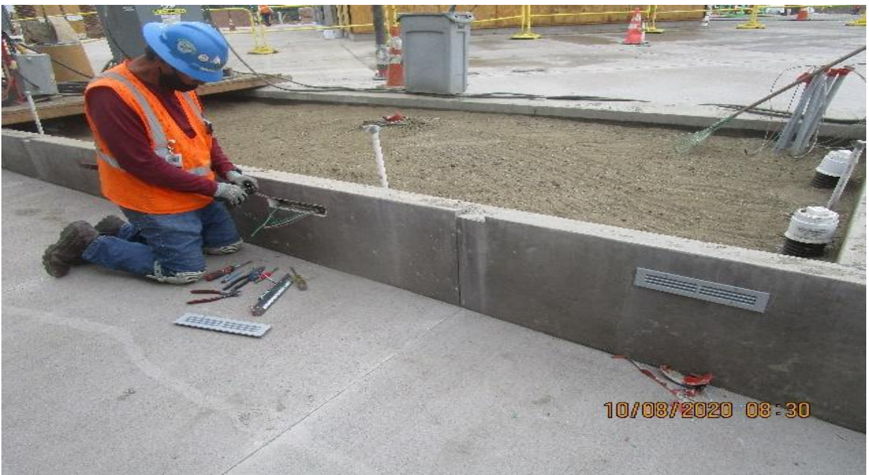
LEIMERT PARK STATION – Installing recessed LED lighting to the entry northern stairs at the plaza.
