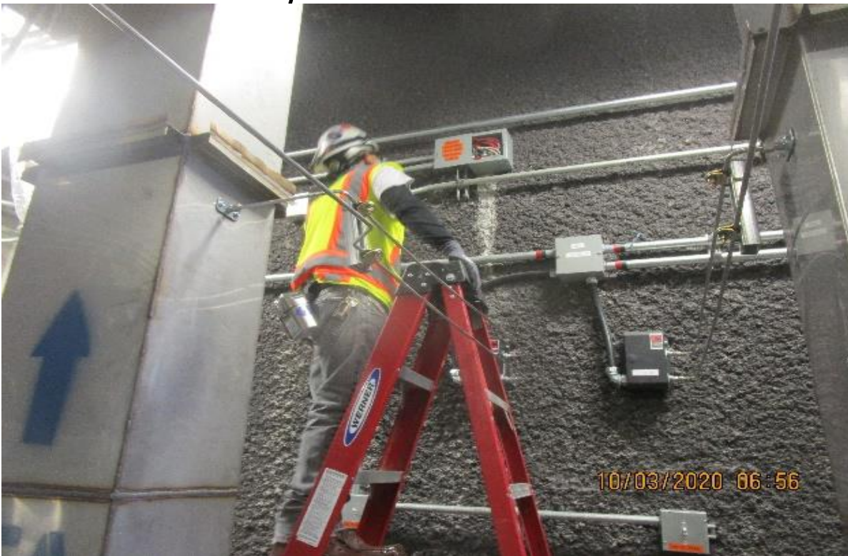
Crenshaw/Vernon – Vernon Mechanical room (S) C114 EF-6-8A & 8B, Pipping 1" GRC & 3/4" seal tight for FSD limit switch control wiring.
