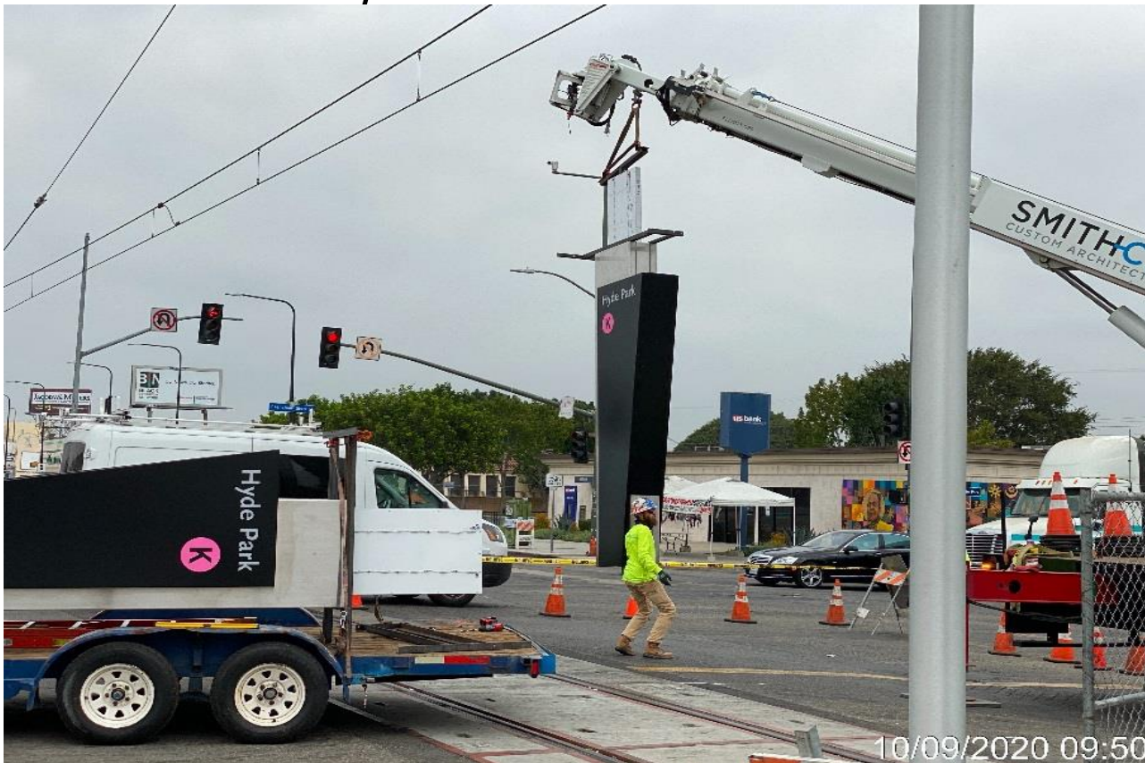
HYDE PARK STATION – Installing the North Grand Pylon sign near Slauson Ave.
