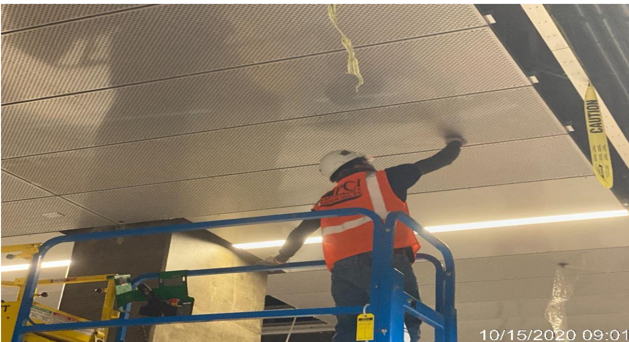
LEIMERT PARK STATION – Continue ceiling panel installation throughout the Free & Paid Area of the concourse level.
