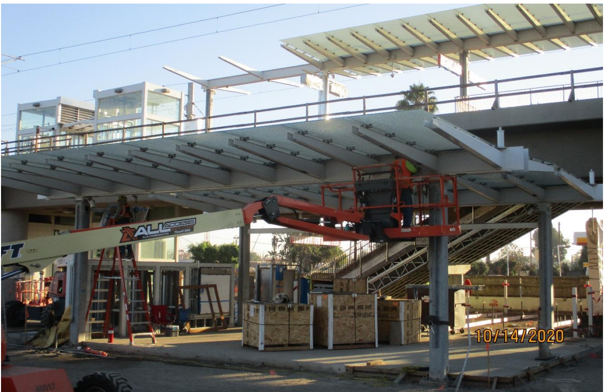
AVIATION/CENTURY- Fire alarm strobe light installation at the Aviation Station ticket kiosk.
