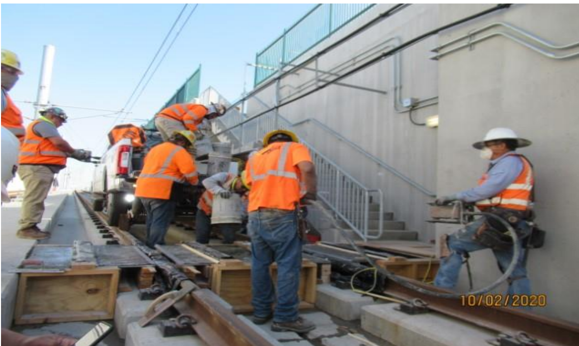
UG1- WSCC placing concrete for newly re-located Emergency Walkway Crossing foundations UG1 NB track STA 56+50 (looking northeast) Rework
