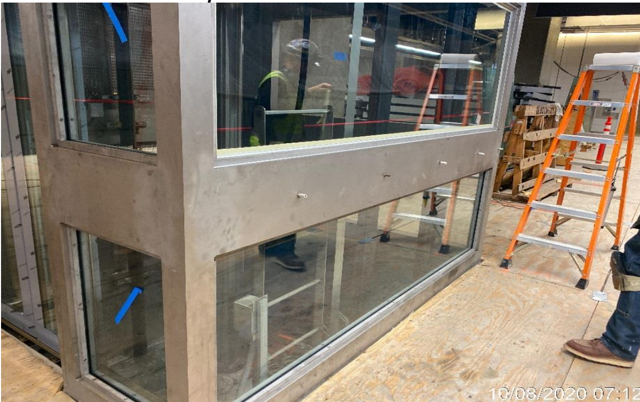
LEIMERT PARK STATION – Continue installing glass tracks for Elevators 3&4 at the platform level.
