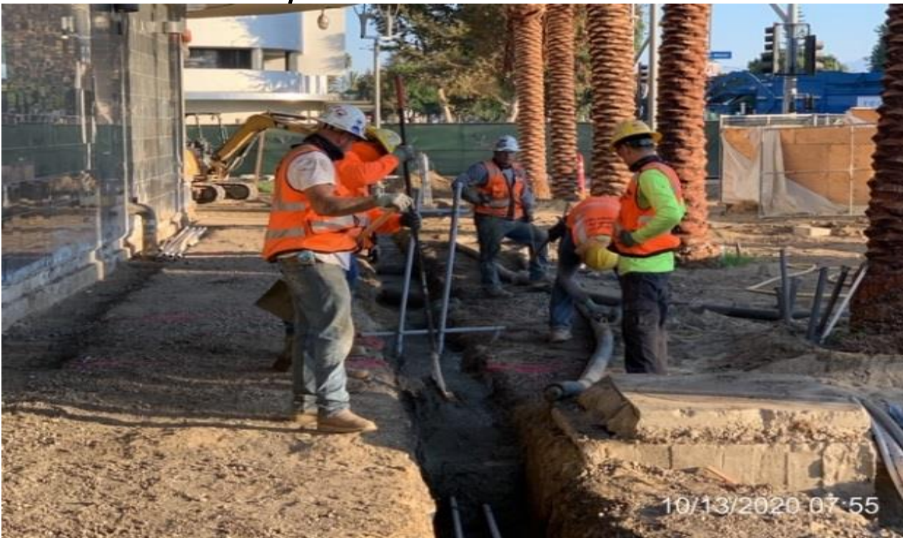
MLK STATION – Placing concrete for the CCTV conduit duct bank for the pedestrian light poles at the plaza level.
