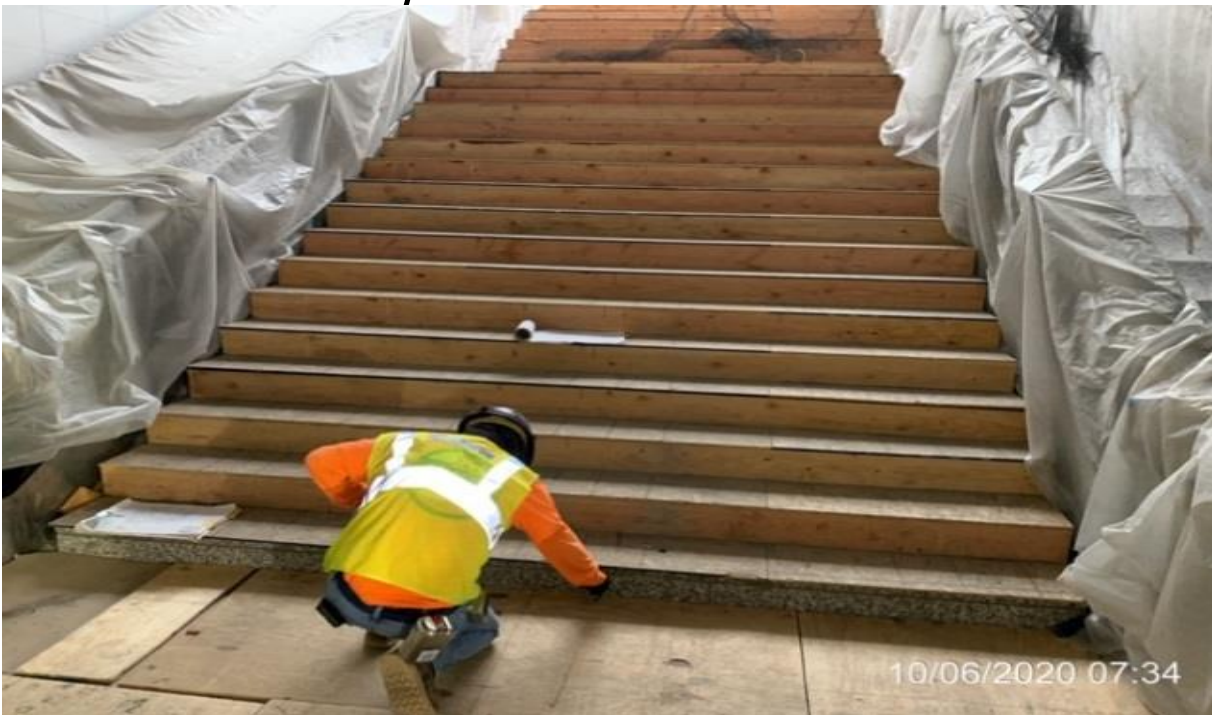
MLK STATION – Laying out for the center handrail of Staircase 1 from plaza to concourse level.
