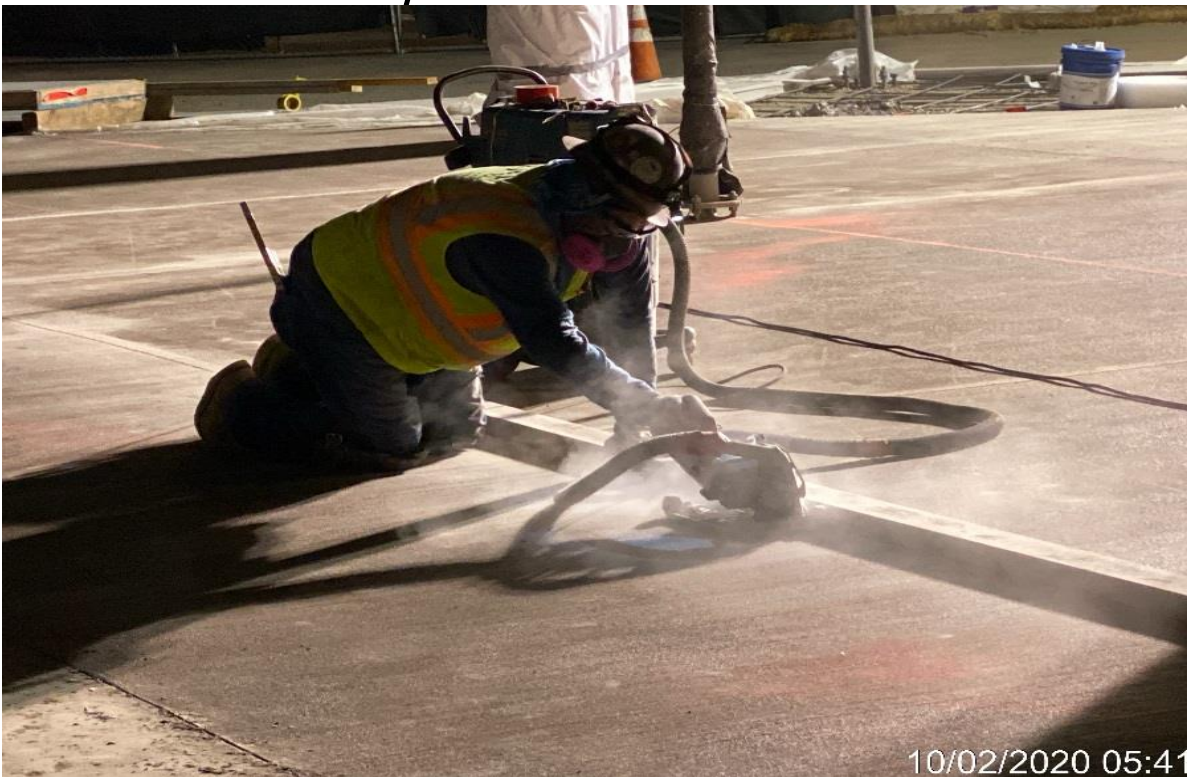
LEIMERT PARK STATION – Continue saw cutting control joints for the architectural topping slab throughout the plaza level.
