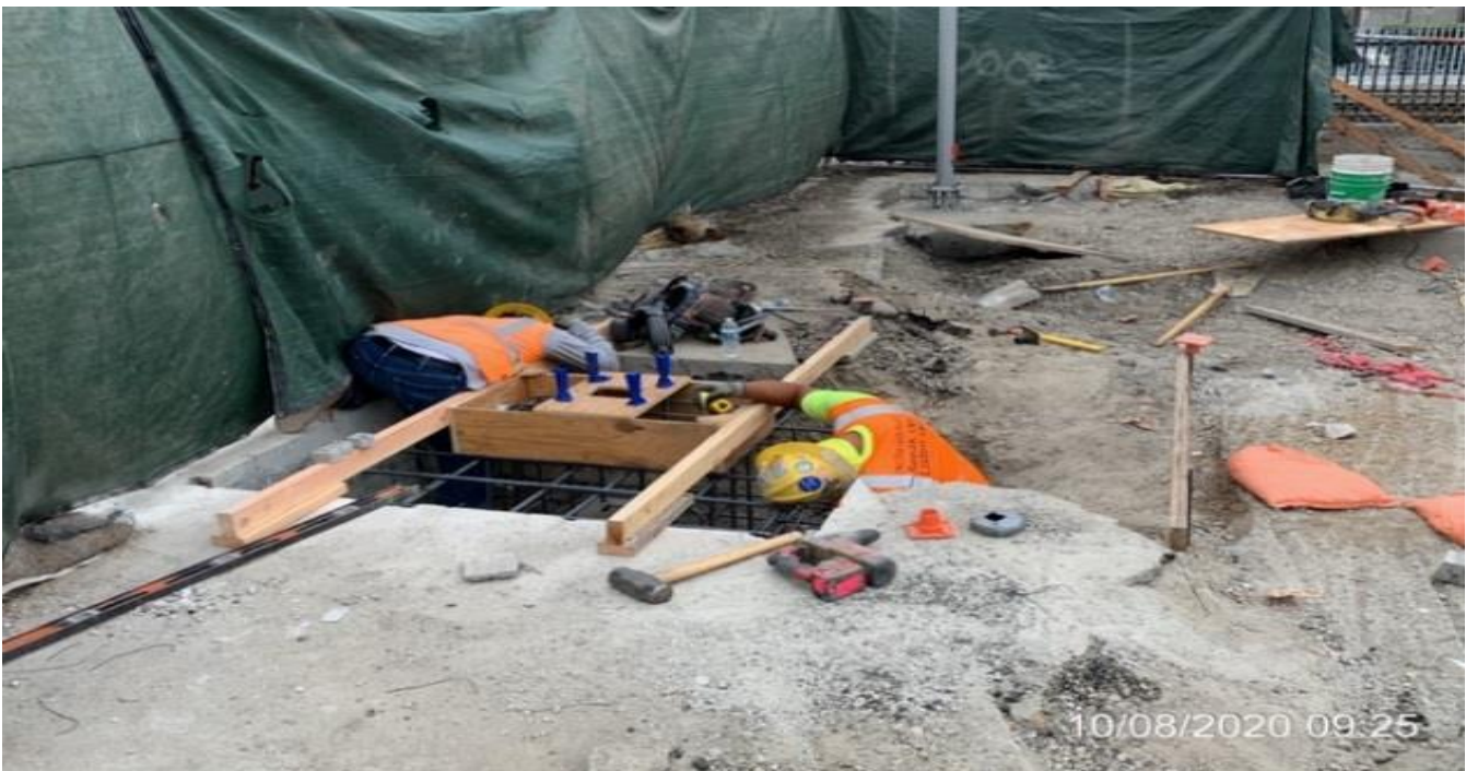
EXPO STATION – Building formwork for the grand pylon foundation footing at the plaza level.
