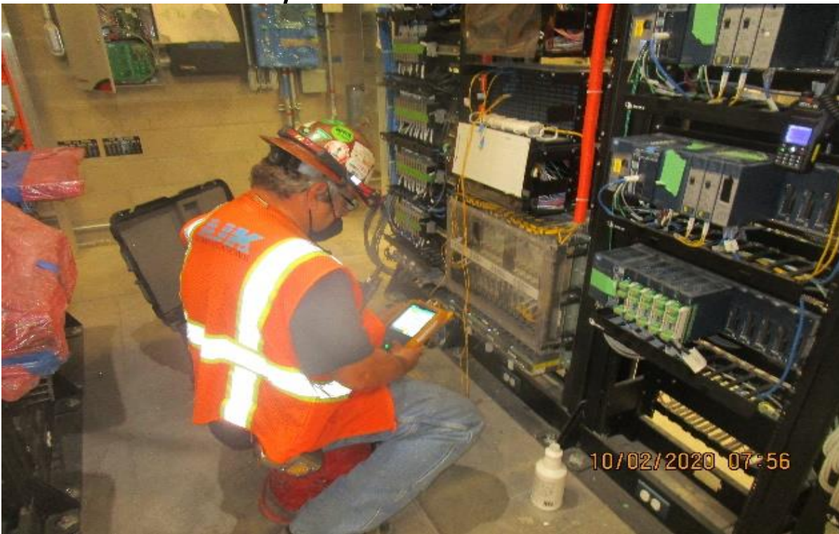
Crenshaw/Vernon – Vernon, TC&C Room C112, CTS Rack testing fiber optic (end to end) to SRI intrusion panel at UG4 Sta 371+05.
