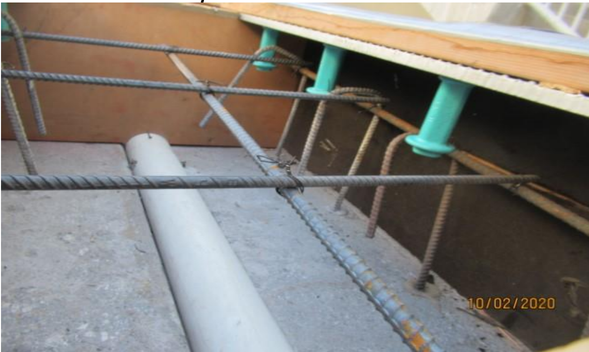
UG1- Emergency walkway crossing foundation showing adequate stirrup & elongated reinforced rebar prior to placing concrete into foundation UG1 NB track STA 56+50 Rework
