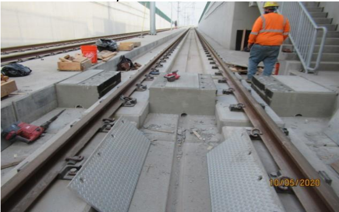
UG1- UG1 NB track STA 56+50 WSCC preparing to bush & butter top of Emergency Walkway Crossing foundations (looking north) Rework.
