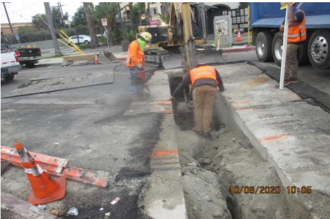
PARK MESA – Excavating for Storm Drain Line F on the northeast corner of Crenshaw Blvd and 60th St.
