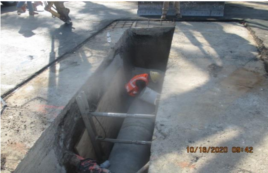
PARK MESA – Installing Storm Drain Line F on northbound Crenshaw Blvd and 60th St.
