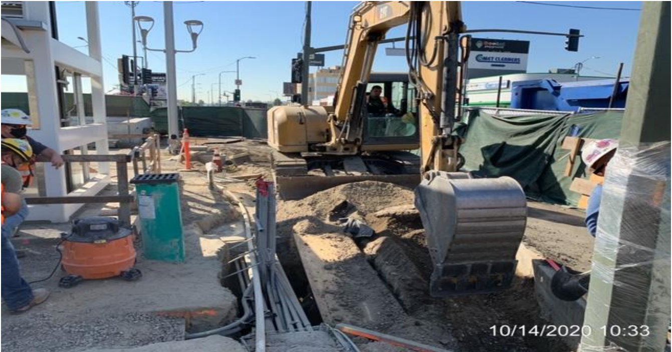
EXPO STATION – Excavating/trenching for the west side bollard foundations at the plaza level.
