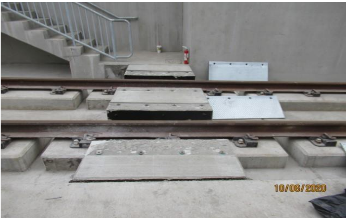
UG1- UG1 NB track STA 56+50 Emergency Walkway Crossing foundation on-going repair work for re-location on crossing (looking east) Rework.
