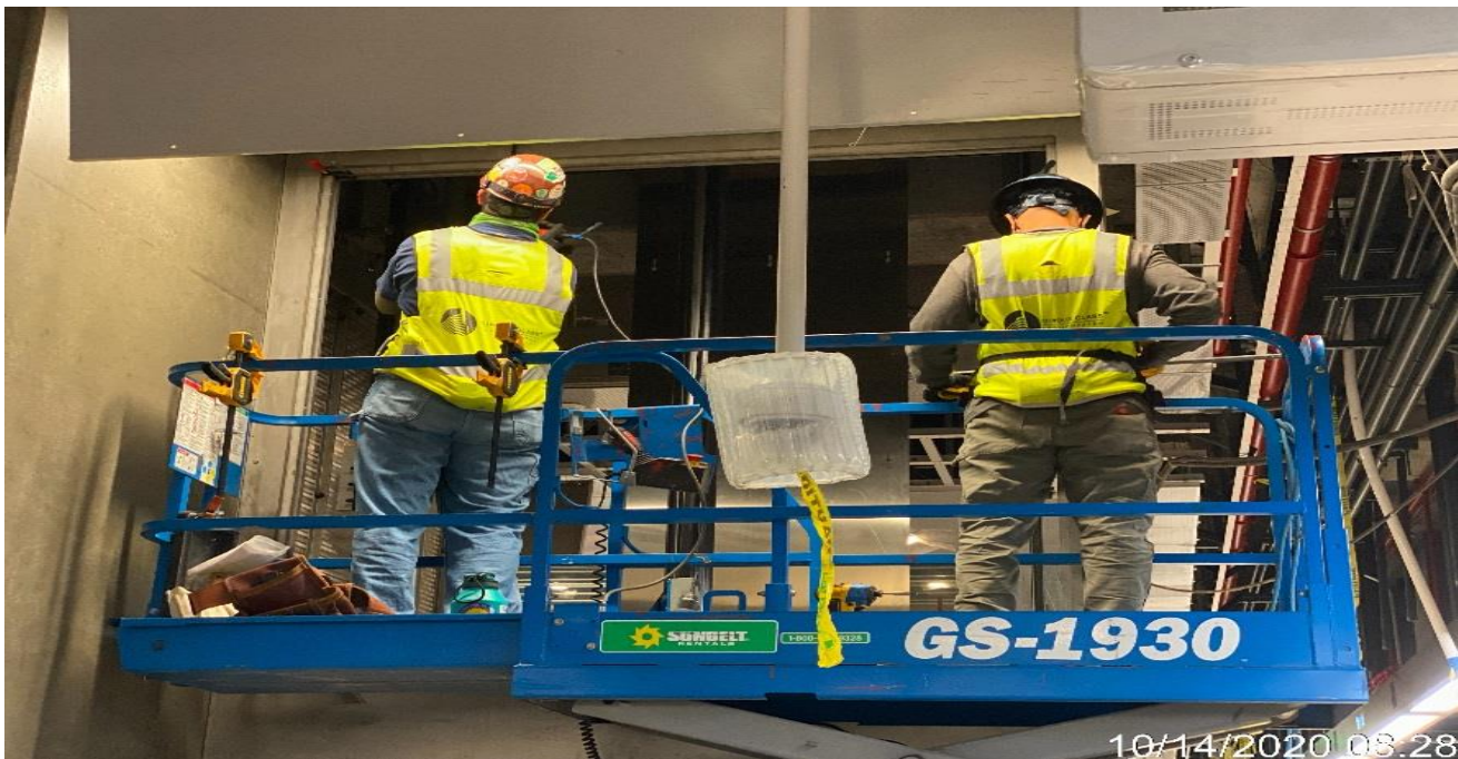
LEIMERT PARK STATION – Continue installing glass tracks for Elevators 3&4 at the platform level.
