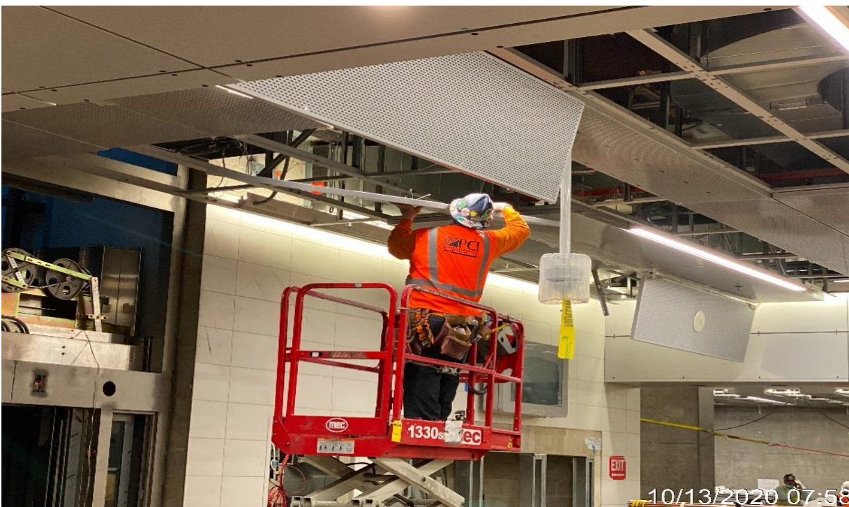
LEIMERT PARK STATION – Continue ceiling panel installation throughout the Free & Paid Area of the concourse level.
