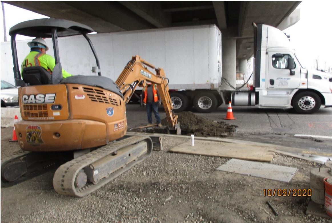
AVIATION/CENTURY- Trenching for the traffic loop stub out at Aviation and Century.
