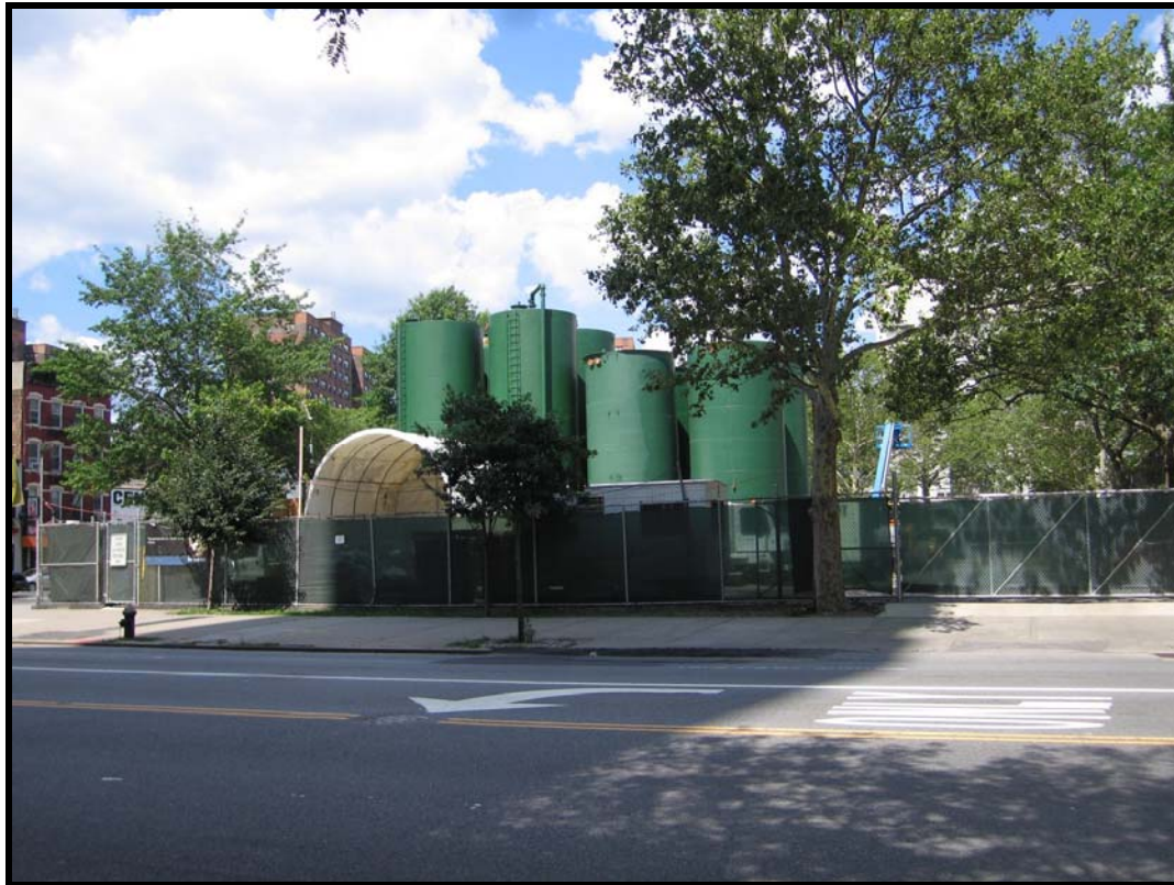
Figure 3-1 - TBM Slurry Plant, New York City Transit, Second Avenue Subway Project, New York, NY
