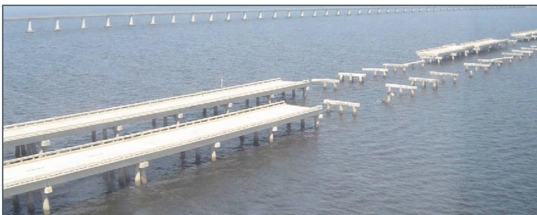
Figure 2.15 Escambia Bay Bridge missing decks after Hurricane Ivan
