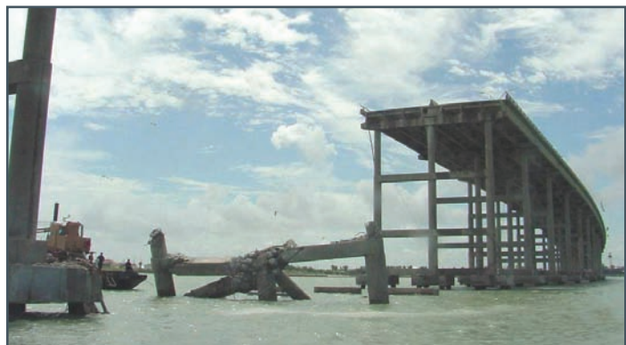
Figure 2.18 Damaged Structure after bent 31 fell on bent 32
