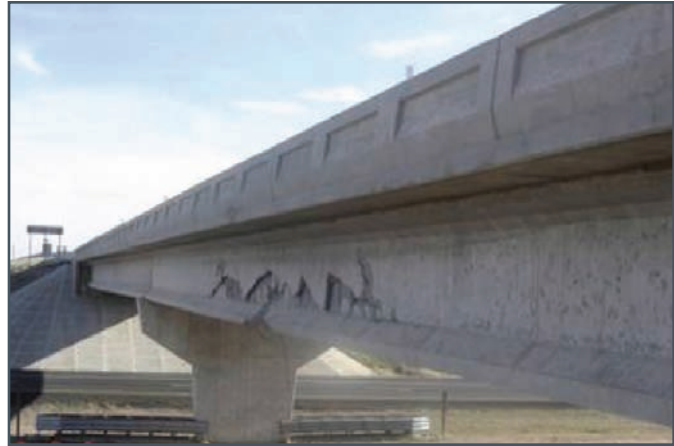
Figure 4.15 I-70 Floy interchange damaged girder
