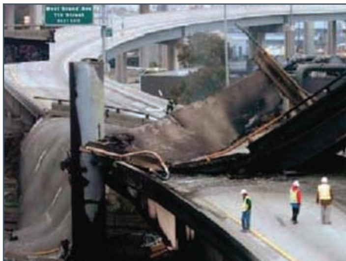
Figure 2.5 MacArthur Maze bridge damage
