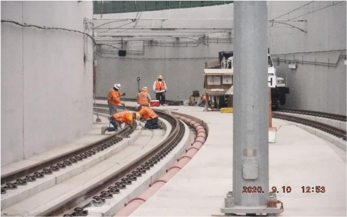
UG3 – STA 279+00 TK#3/SB looking north – NCR-A-111.B – housekeeping after PCC pour and form removal – UG3 (Victoria)
