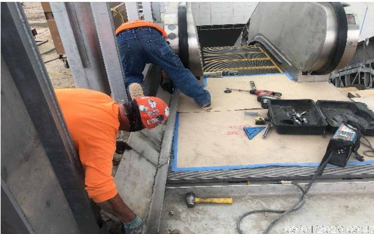
EXPO STATION – WSCC ironworkers installing bent plates at escalator #1 and #2 top landing.
