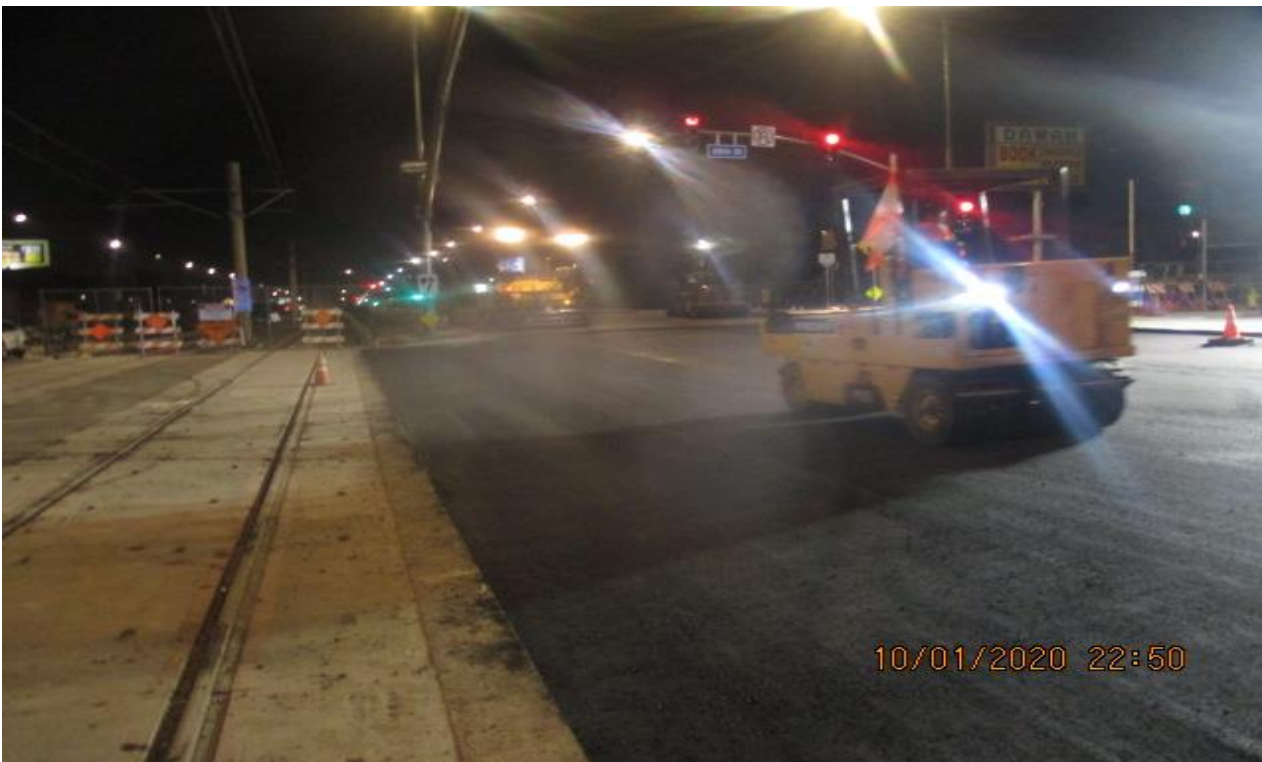
PARK MESA – Placing asphalt concrete for Lanes 1&2 of southbound Crenshaw Blvd and 48th St.
