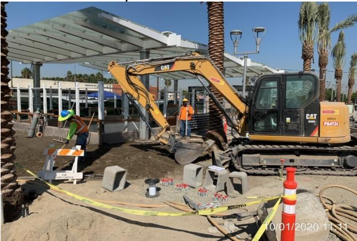
EXPO STATION – Excavating/grading near the main entrance canopy at the plaza level.
