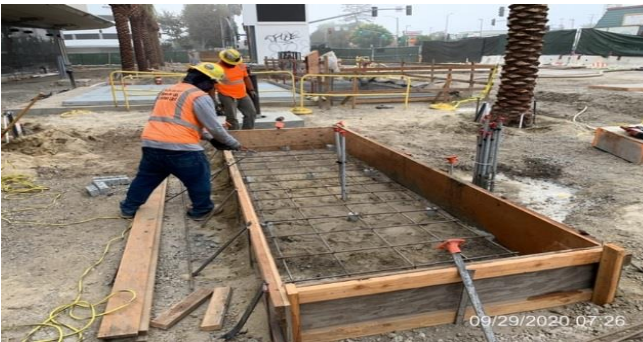
MLK STATION – Building formwork for the north map case at the plaza level.
