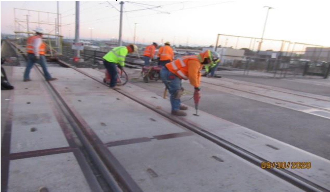
Arbor Vitae- WSCC preparing grade crossing panels to be removed at Arbor Vitae for damaged rail replacement (looking northeast) Rework RFI-01499
