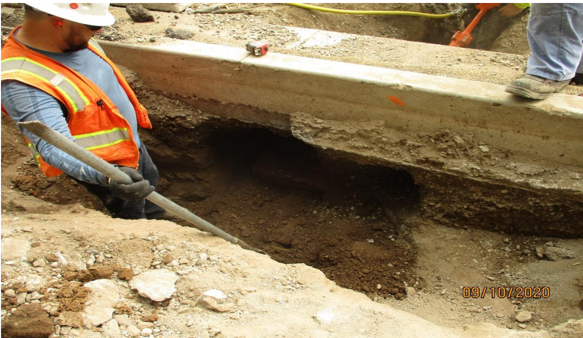
104 th street- Abandoned pipe line that conflicts with the traffic signal conduit on the NW corner of Aviation and Century.
