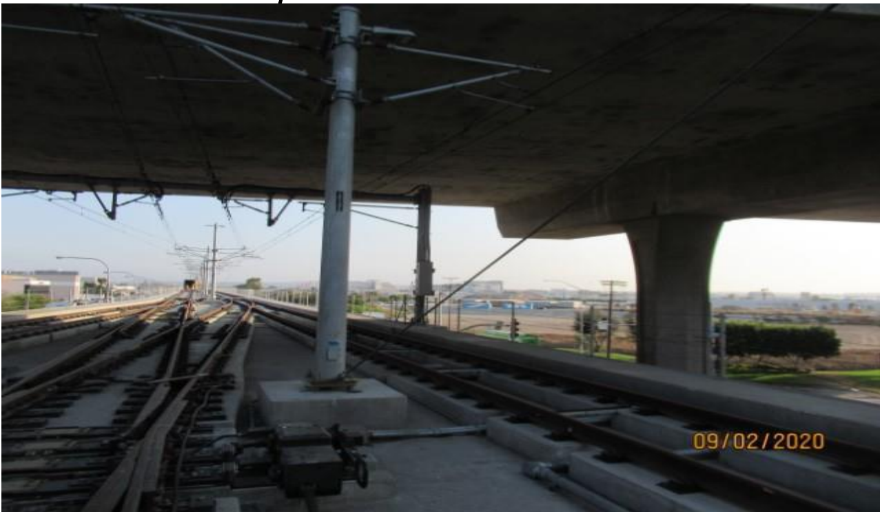
Guideway- OCS pole 1014E at GL Wye Down guy wire still in place over Switch Machine for MPF 3X-ING (looking northeast)
