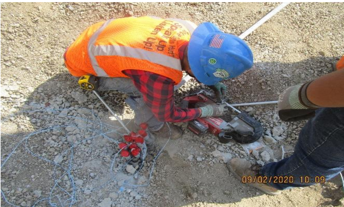
MLK STATION – MLK Plaza, begin to relocate plaza pedestrian lighting stubbed up PVC conduit for embedded PB GL's 16/A.5
