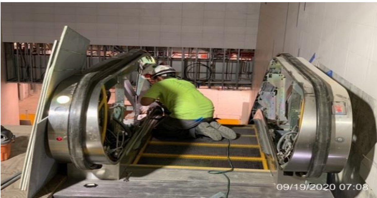
LEIMERT PARK STATION – Continue performing start-up and energization work for all 6 Escalators inside the station.
