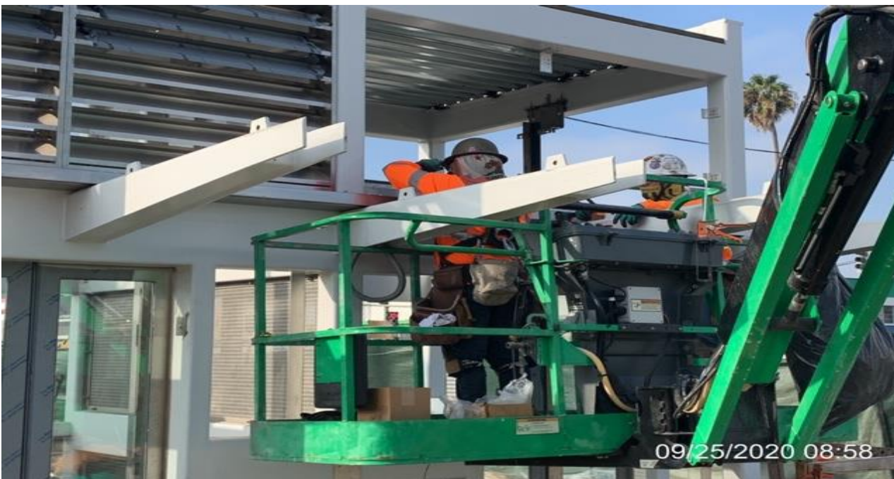
EXPO STATION SITE – Continue installing gutters and louvers to Elevators 1&2 at the plaza level.
