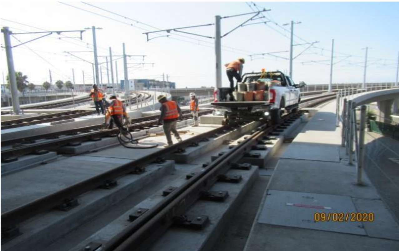
Guideway- LKC & HCC installing & adjusting connecting rods for 10ERH XO at GL Wye (switch point repair) (looking northeast) Rework
