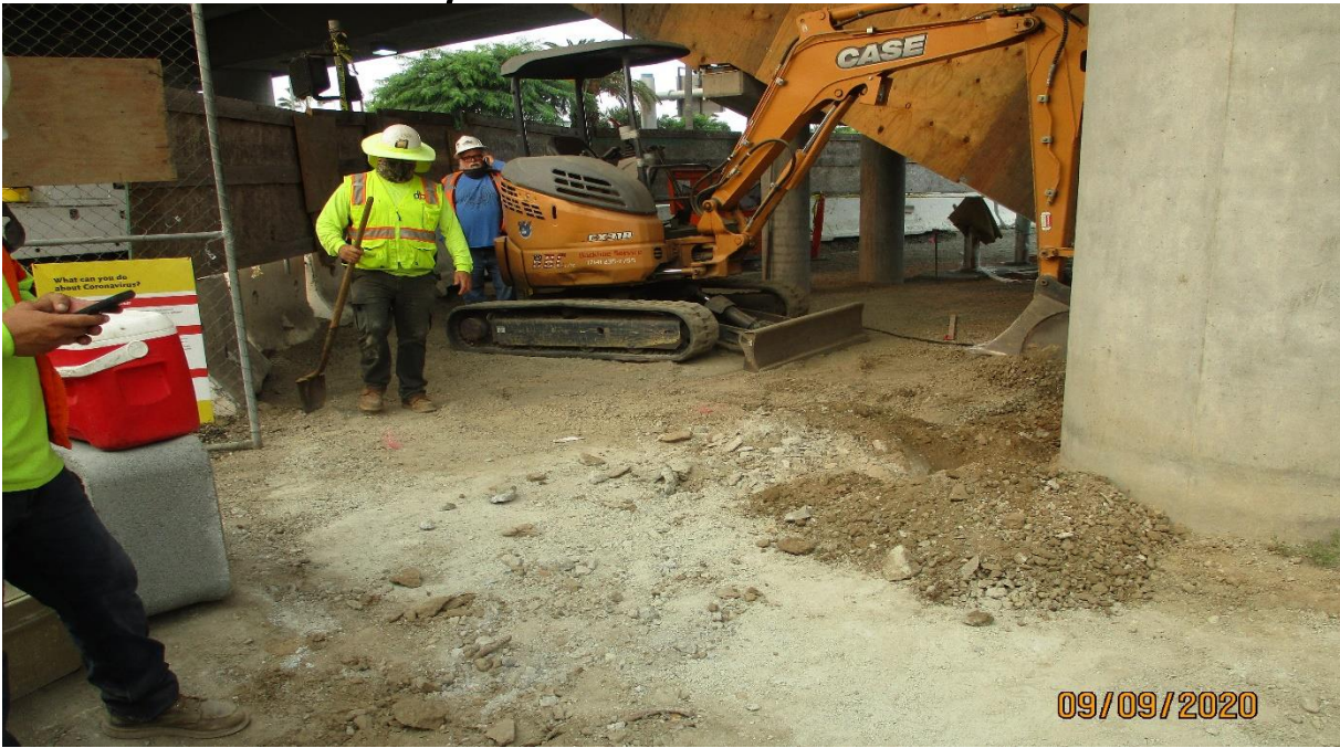
AVIATION/CENTURY- Trying to trench through slurry backfill for traffic signal conduit at the NWC corner of Aviation and Century.
