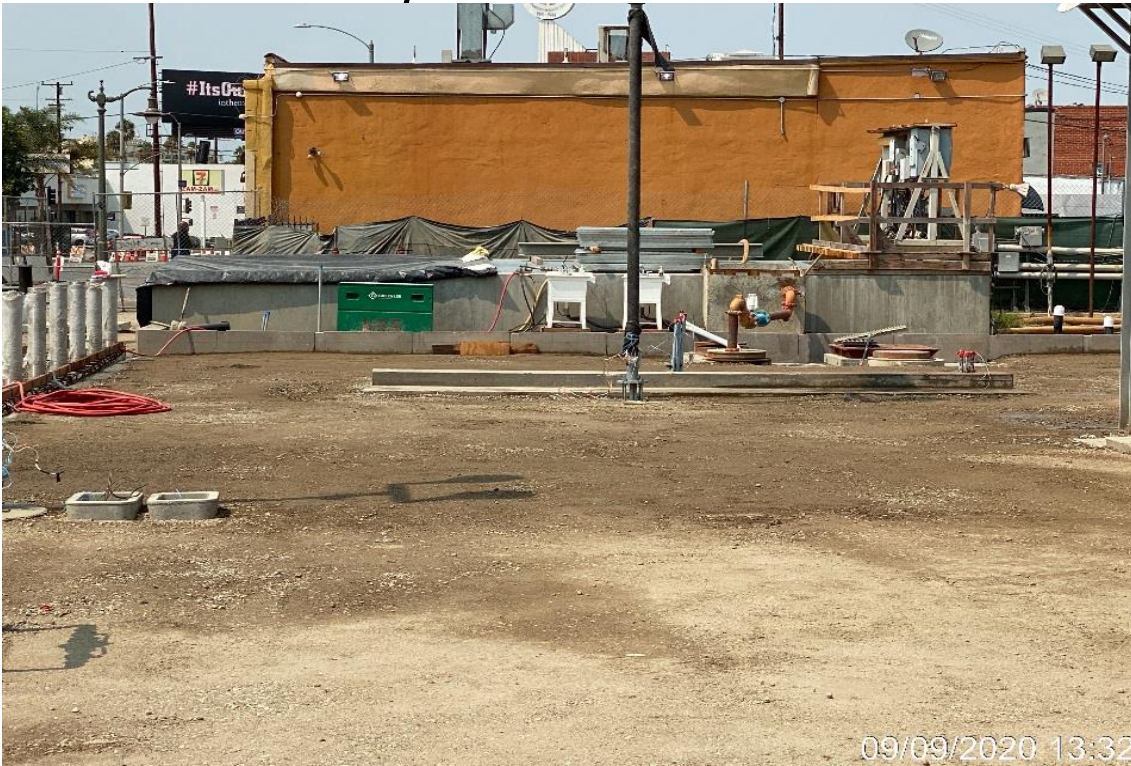
LEIMERT PARK STATION – Setting forms for concrete placement of the architectural topping slab throughout the plaza level.
