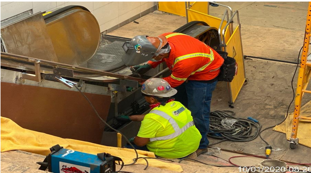
LEIMERT PARK STATION – Continue welding brackets for handrail installation from the intermediate landing to the concourse level.
