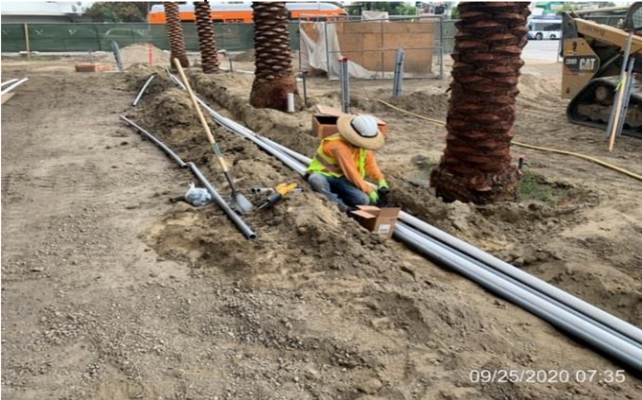
MLK STATION – Laying out irrigation lines at the northwest end of the plaza level.
