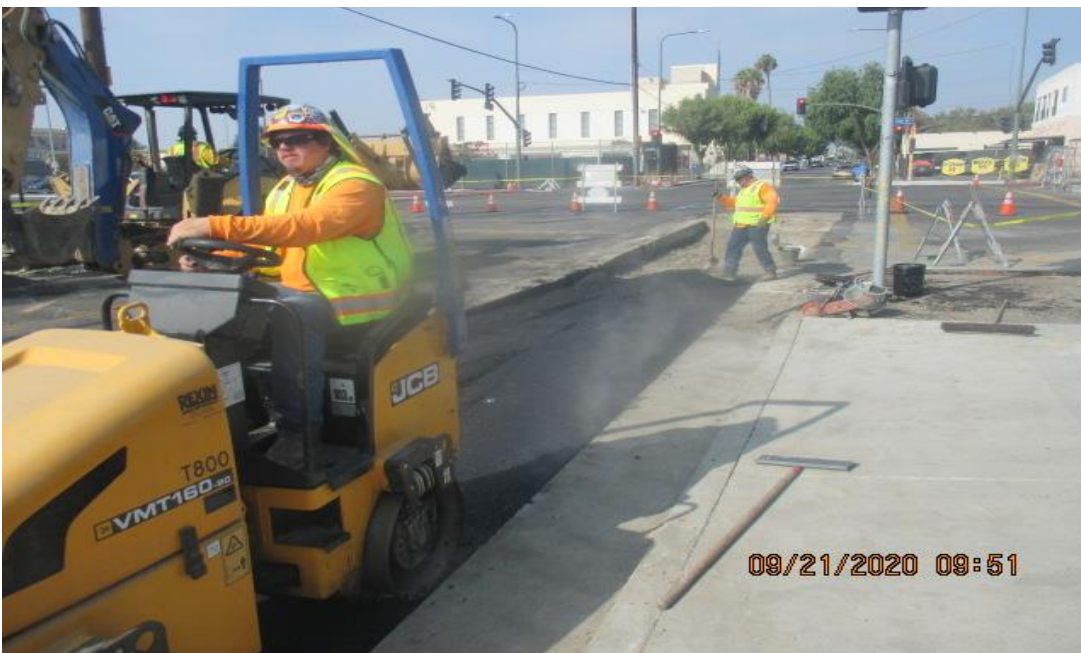
PARK MESA – Continue placing asphalt concrete on northbound Crenshaw Blvd and 60th St.
