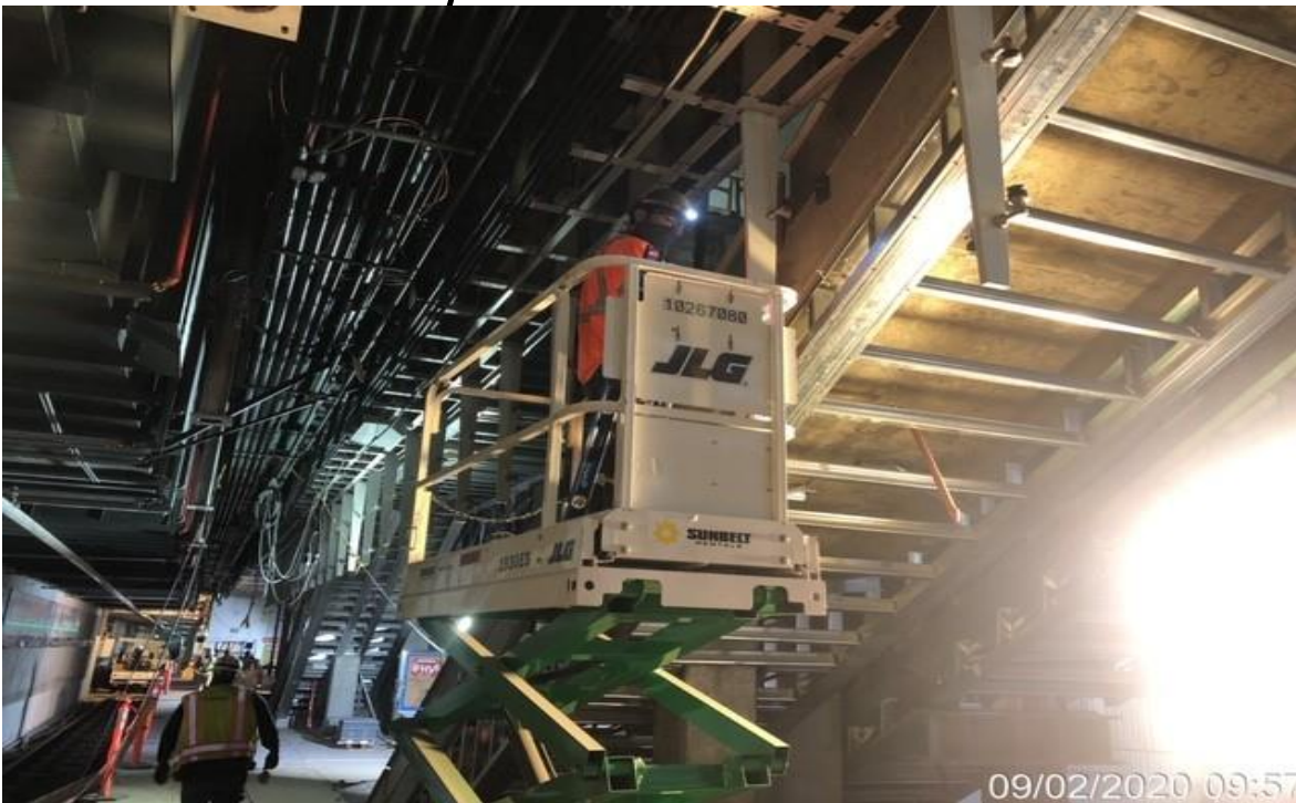
EXPO STATION – VNSM doing layout for stainless steel cladding for soffit and sides of escalators and stairs.
