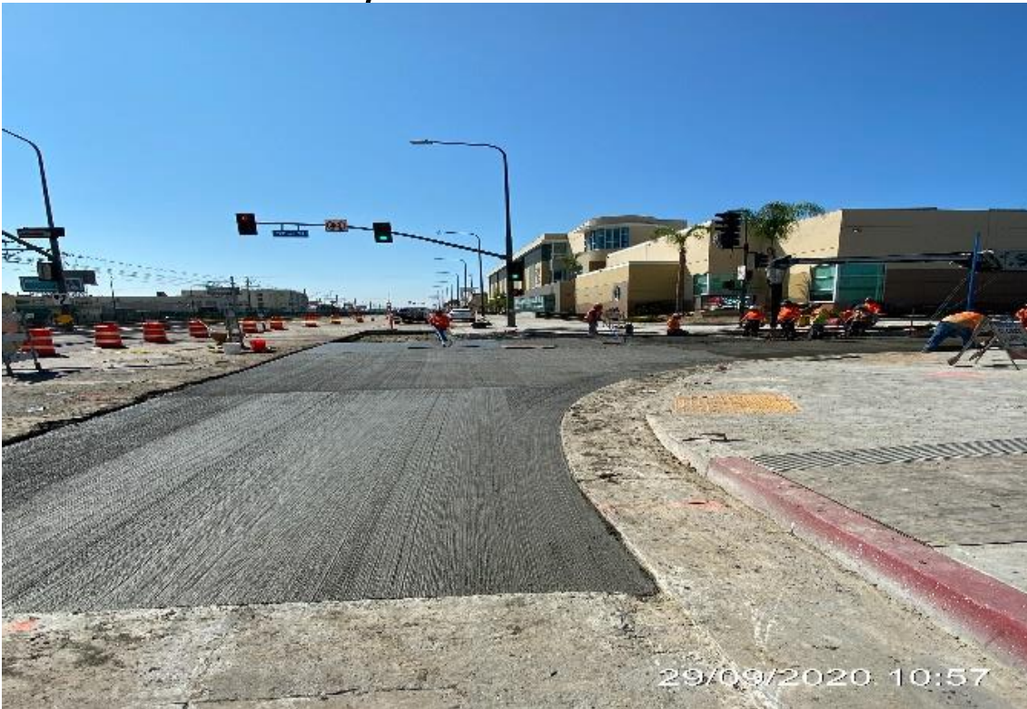
PARK MESA – Continue placing concrete along the southbound lane of Crenshaw Blvd and 52nd St.
