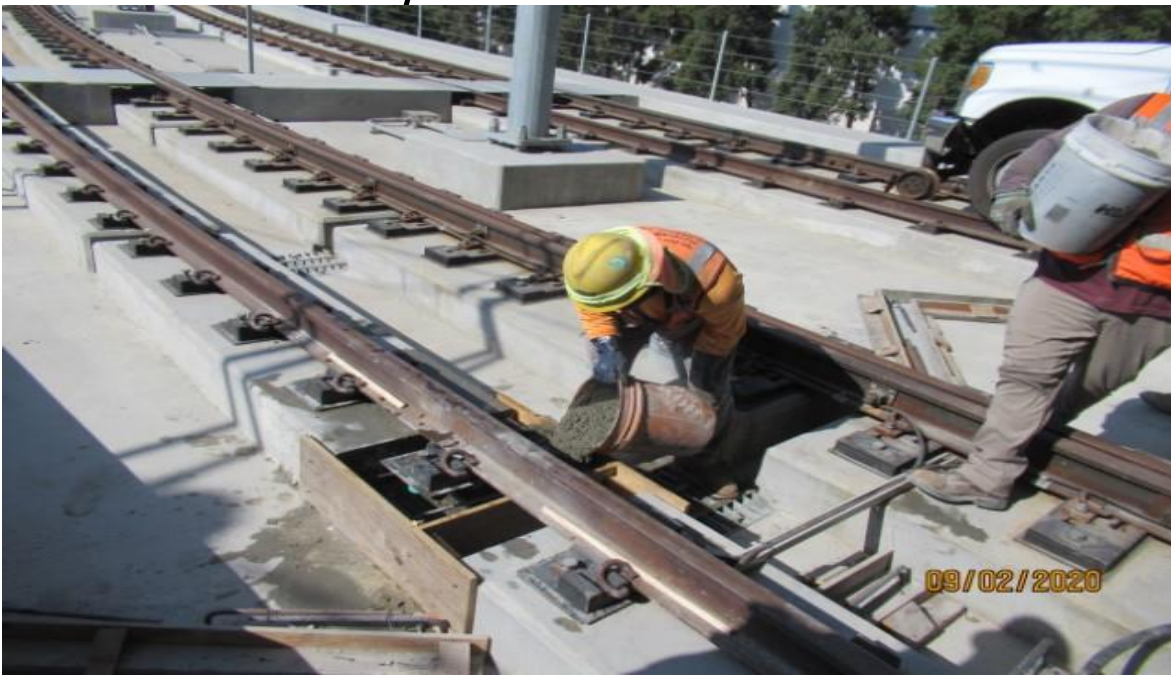
Guideway- WSCC using 5-gal. buckets to place concrete into end of plinth on NBW track GL Wye, Rework for NCR-A 111-B case 4
