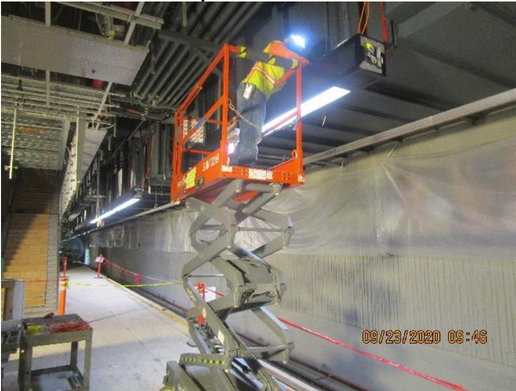
MLK STATION – Continue installing edge light fixtures to the down stand support posts on the north and southbound platform level.
