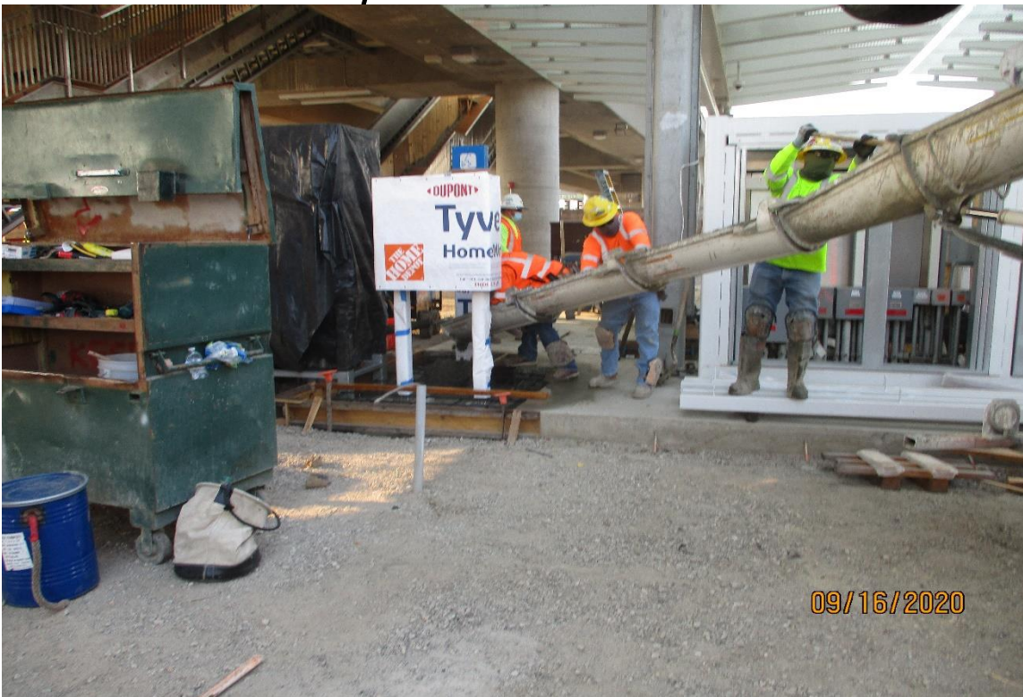
104 th street- Placing concrete for the IFF pad at the Aviation Station.
