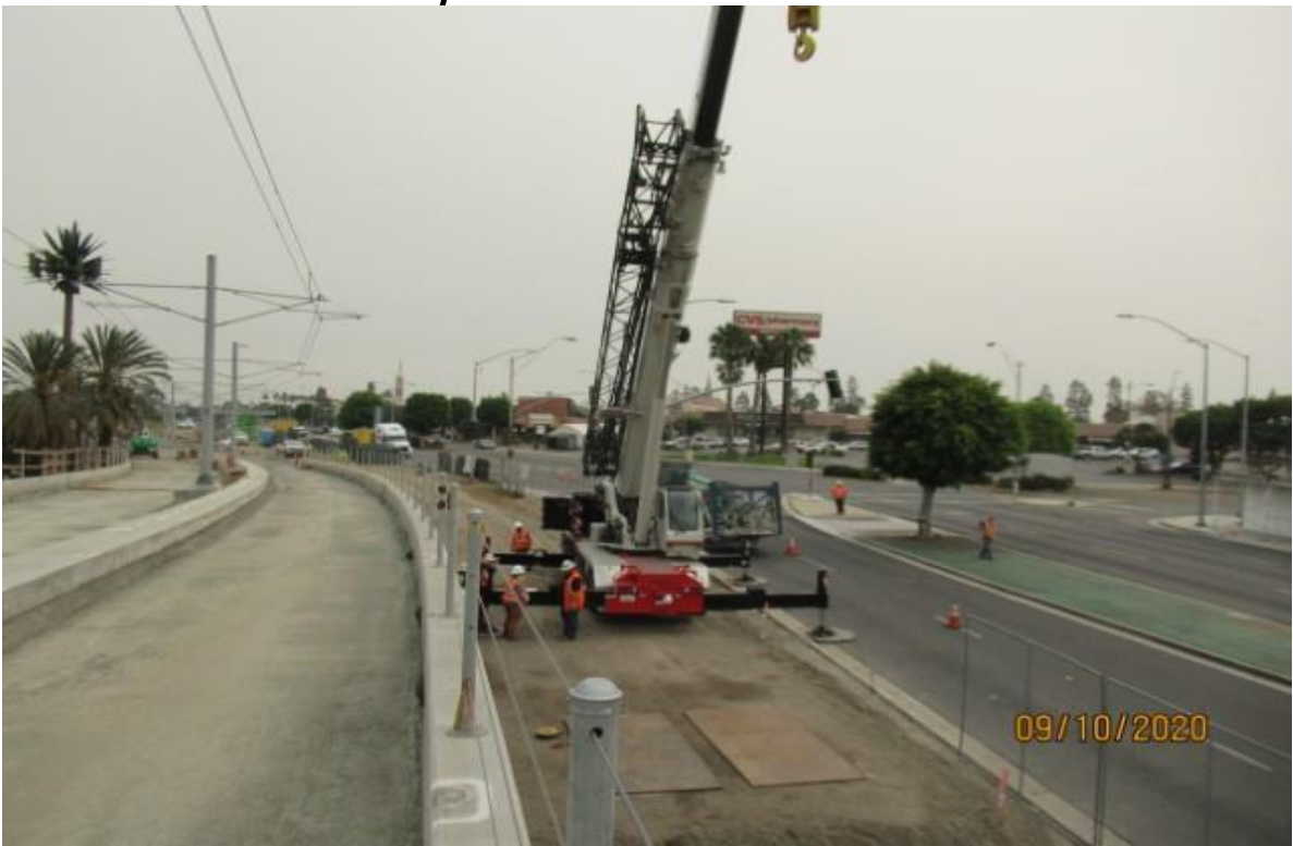
La Brea – La Brea wall 202 WSCC sub-contractor mobilizing & setting up Crain for repair work to be done (looking north) Rework
