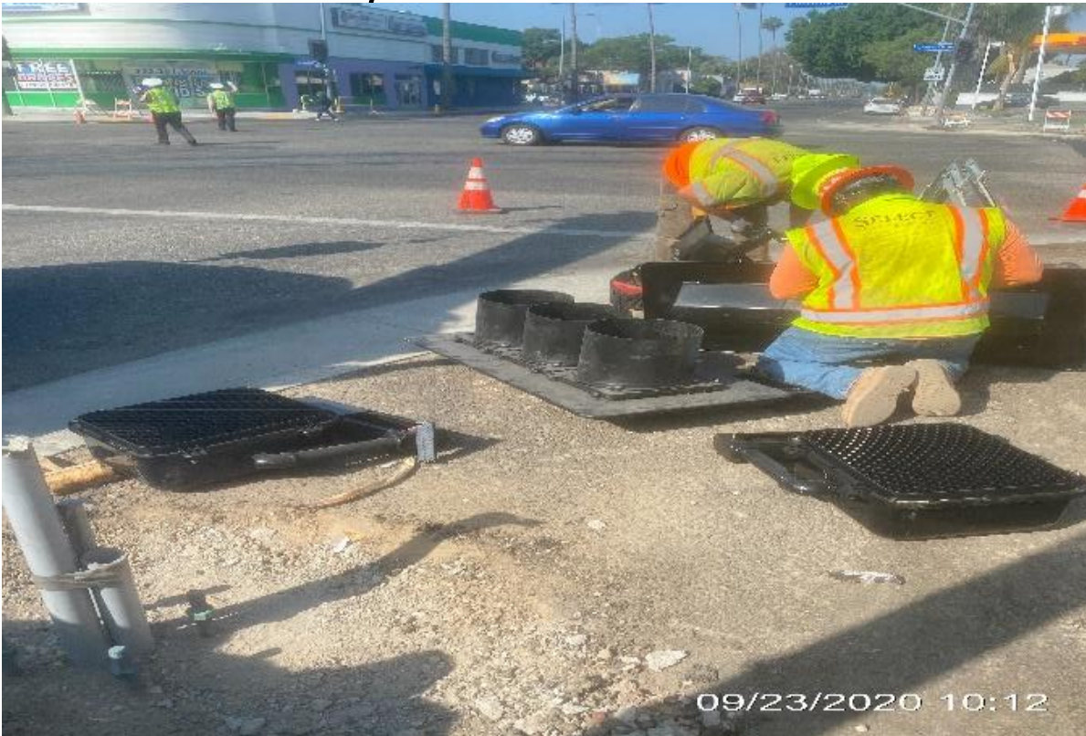
EXPO STATION– Assembling traffic signal light pole for installation on the northeast corner of Obama Blvd and Crenshaw Blvd.
