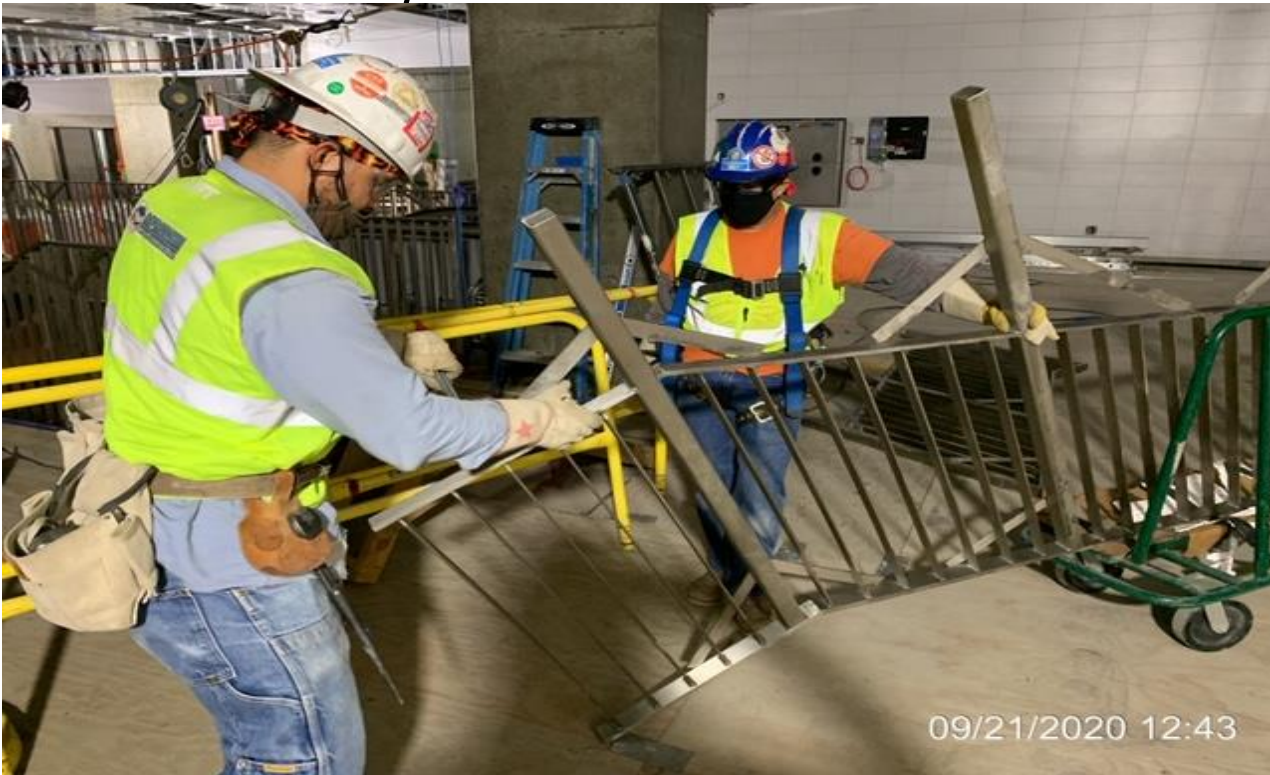
MLK STATION – Installing guardrails around the opening entrance of Staircase #3 and Escalator #4 at the concourse level.
