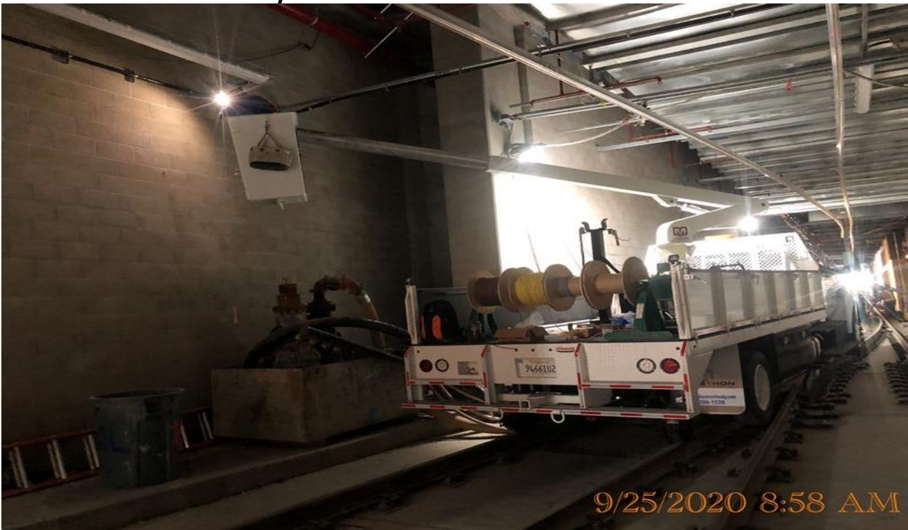
EXPO STATION – Continue installing supports and fixtures for the crossover lighting at the invert level.
