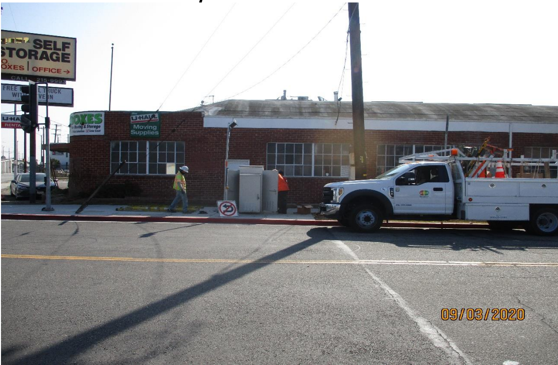
Hindry – Traffic signal controller wiring at Hindry and Florence.
