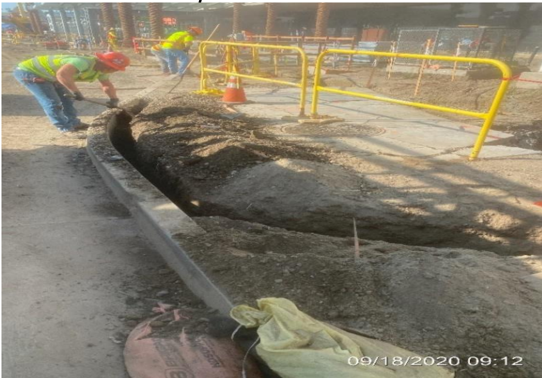
MLK STATION – Continue trenching for street light conduit installation along the plaza curb.
