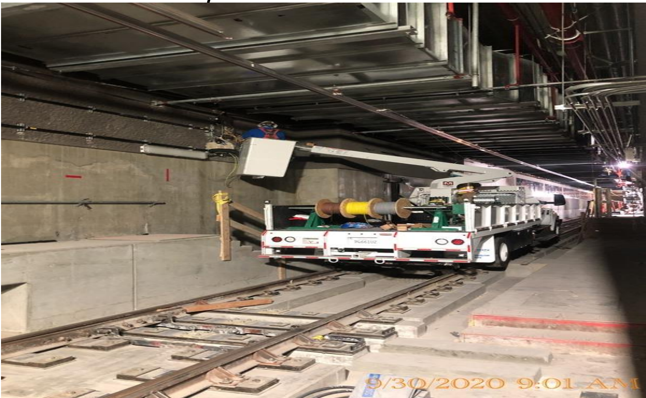
EXPO STATION – Continue installing supports and fixtures for the crossover lighting at the invert level.
