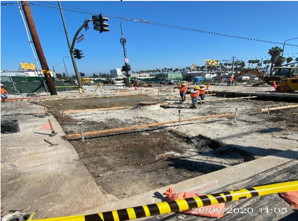
PARK MESA – Setting formwork in preparation for concrete placement along the southbound lane of Crenshaw Blvd and 48th St.
