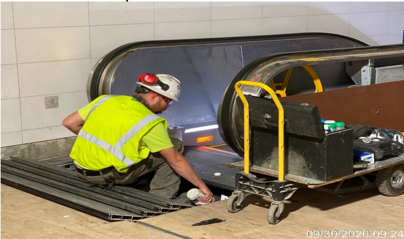
LEIMERT PARK STATION – Continue performing start-up and energization work for all 6 Escalators inside the station.
