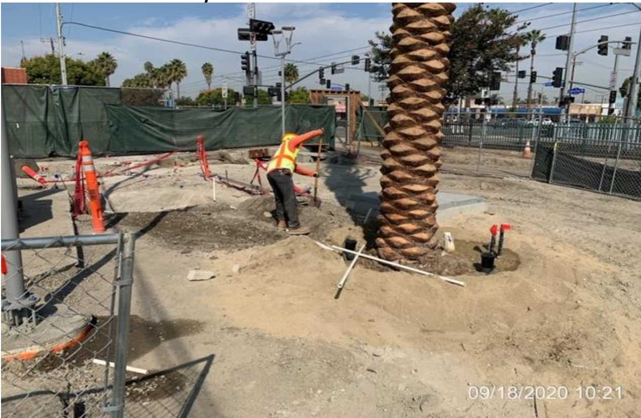
EXPO STATION – Continue excavating for irrigation installation along the north plaza level..
