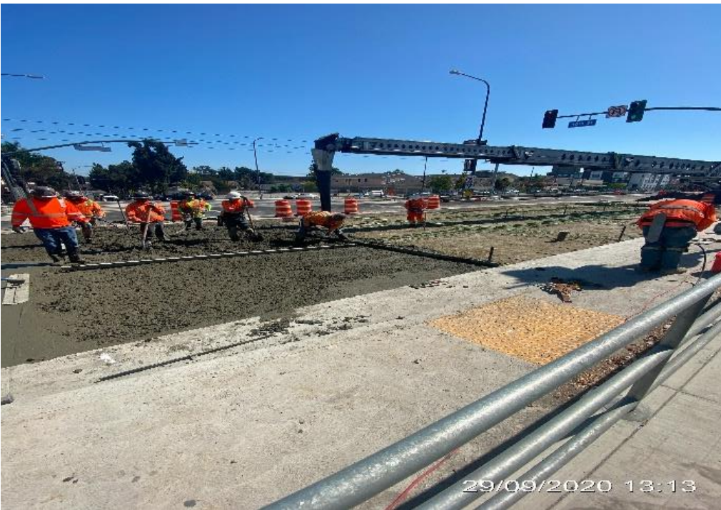
PARK MESA – Continue placing concrete along the southbound lane of Crenshaw Blvd and 50th St.
