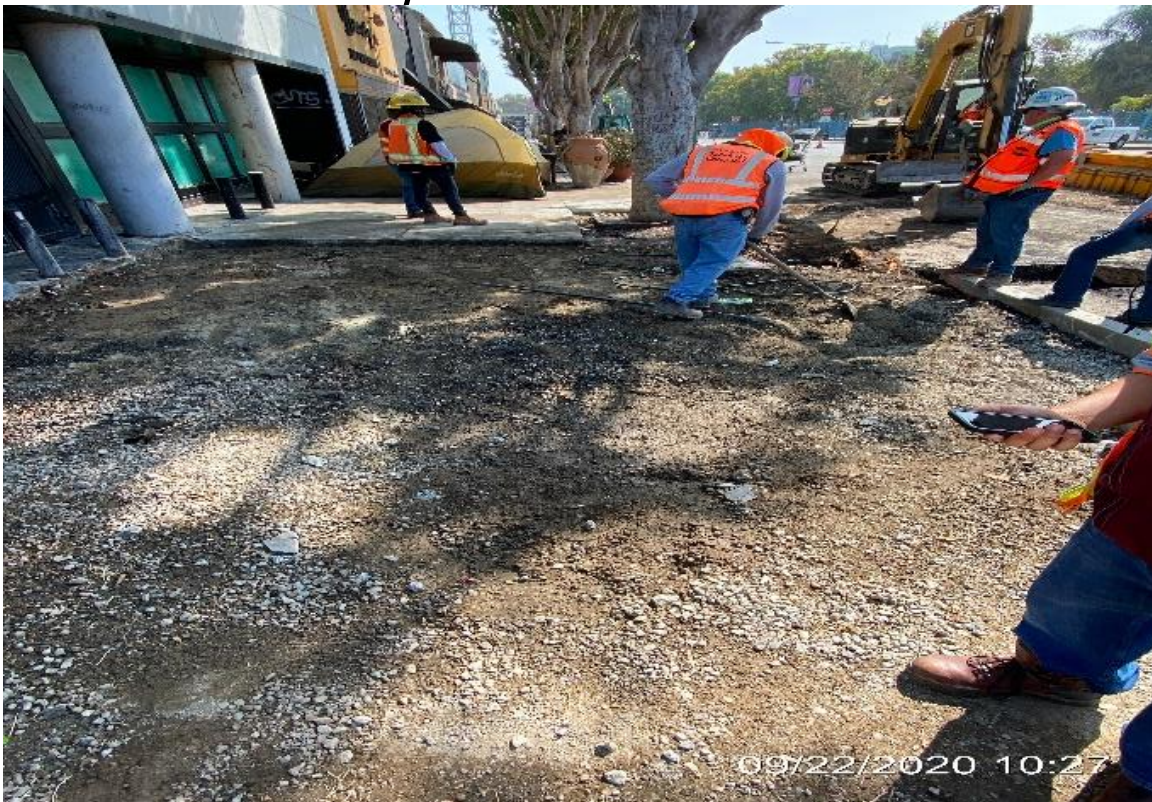
LEIMERT PARK STATION – Excavating/grading sidewalk for restoration on the far northeast corner of Crenshaw Blvd and 43rd Pl.
