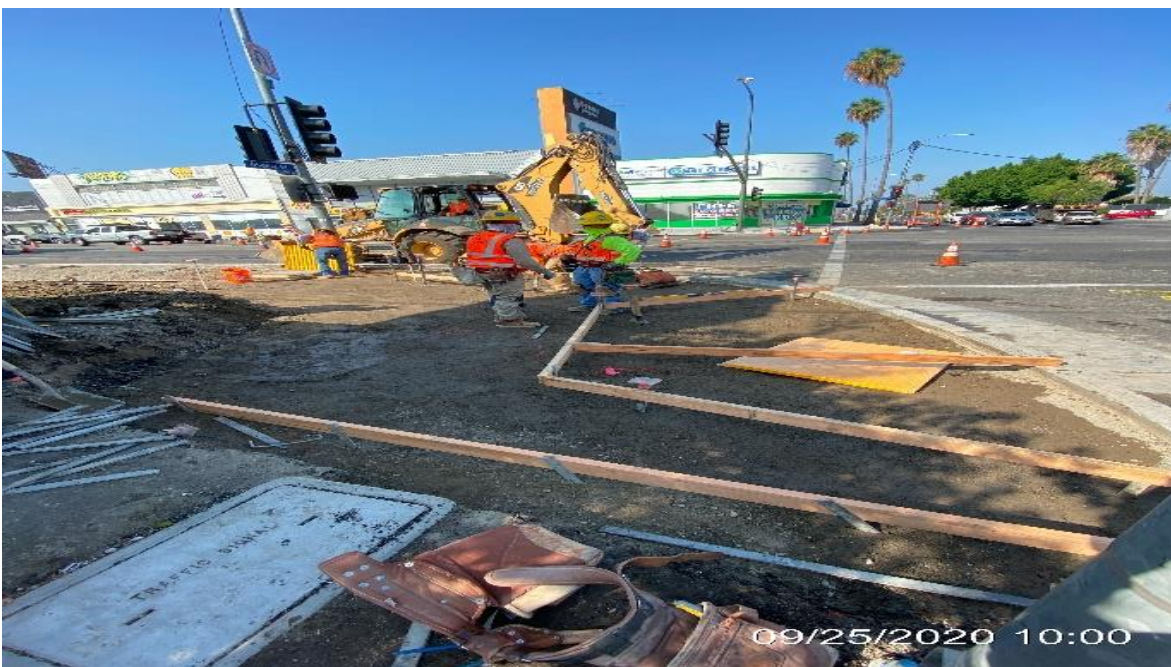
EXPO STATION– Placing forms for new ADA ramp installation on the southeast corner of Obama Blvd and Crenshaw Blvd.
