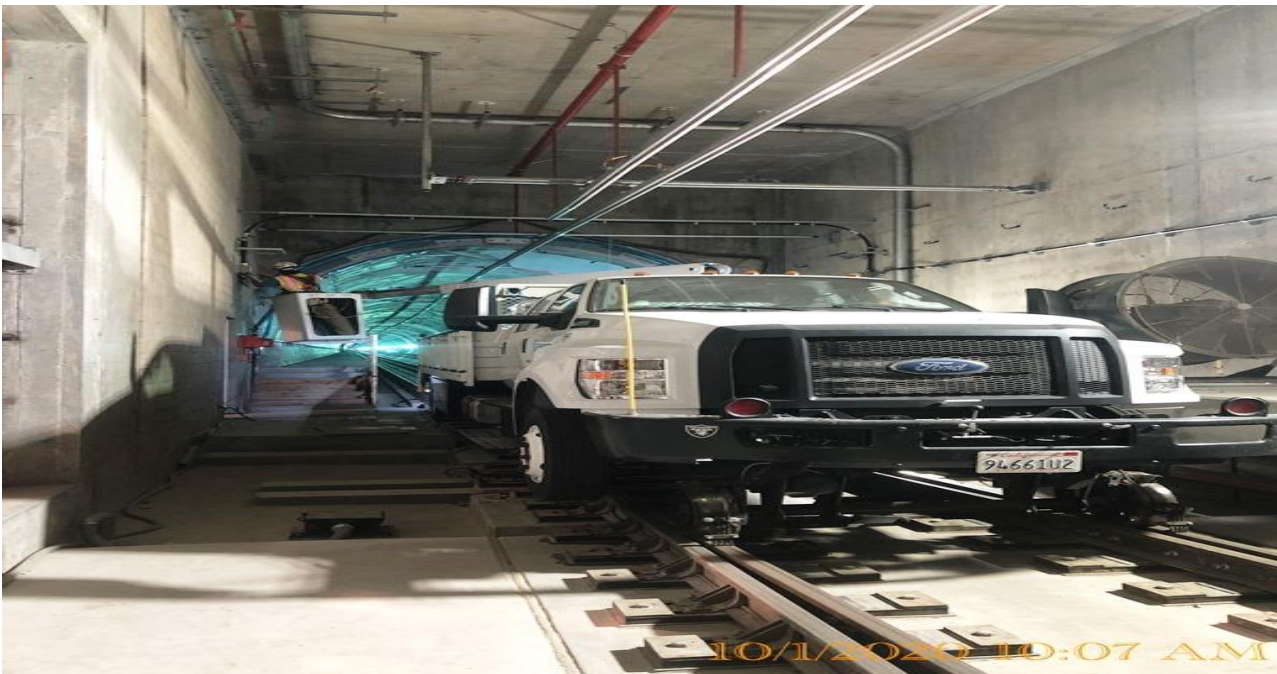
EXPO STATION – Continue installing supports and fixtures for the crossover lighting at the invert level.
