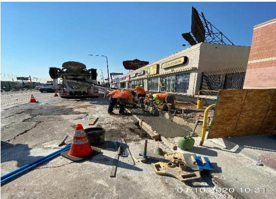
PARK MESA – Placing concrete for the new curb/gutter installation along SB Crenshaw Blvd between 54th and 57th St.
