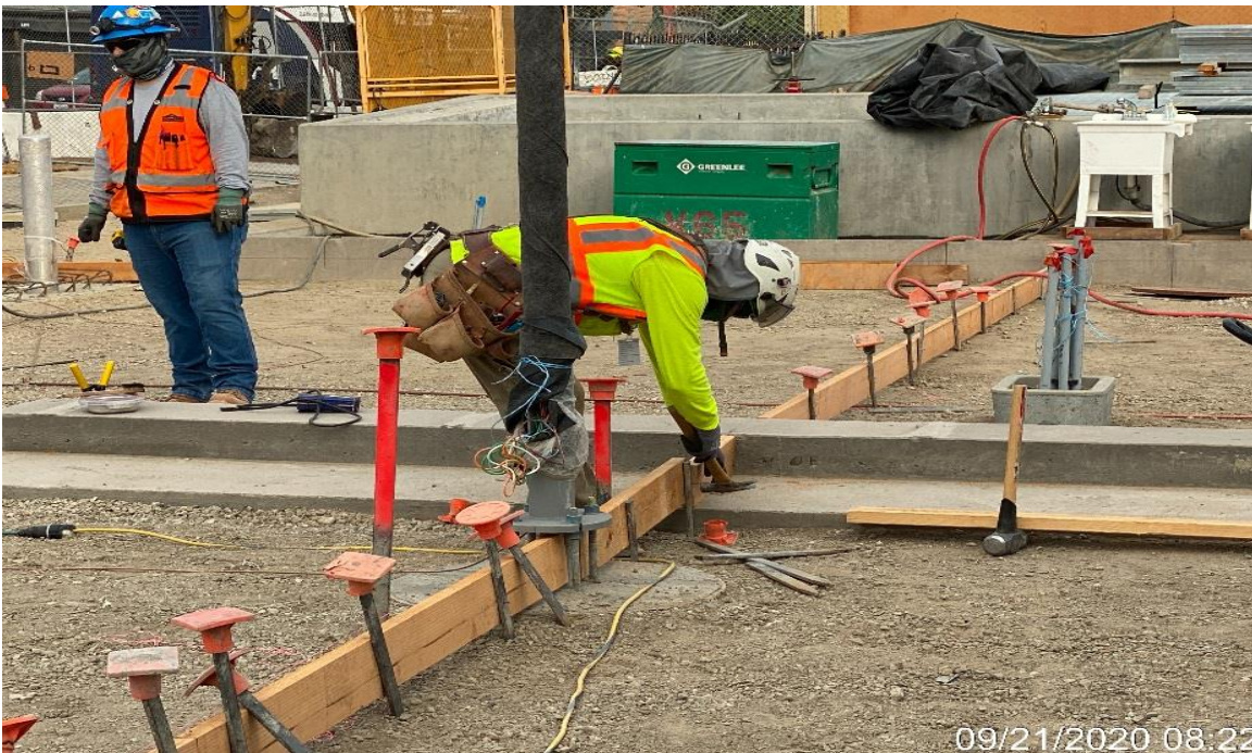
LEIMERT PARK STATION – Continue setting forms for concrete placement of the architectural topping slab throughout the plaza level.
