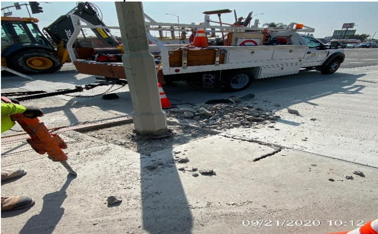
MLK STATION – Removing pedestrian light poles foundation for new installation near the northwest corner Stocker St and Crenshaw Blvd.
