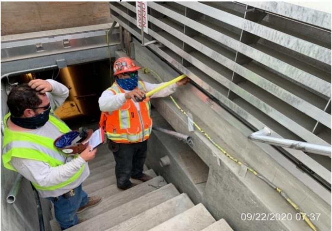
EXPO STATION SITE – Installing galvanized handrails to Emergency Exit Stair #3 at the plaza level.
