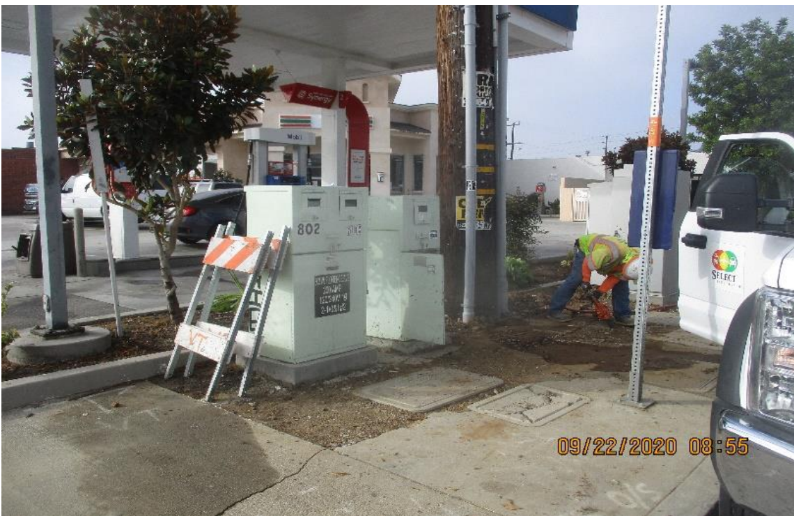
Hindry – Select Electric Remove old controllers at S/WCOR of La Cienerga and Florence..
