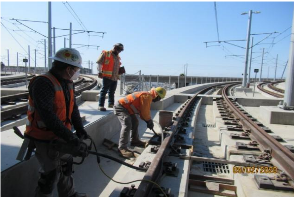
Guideway- WSCC vibrating concrete in repaired plinth on NBW at GL Wye (looking south) Rework for NCR-A 111-B case 4
