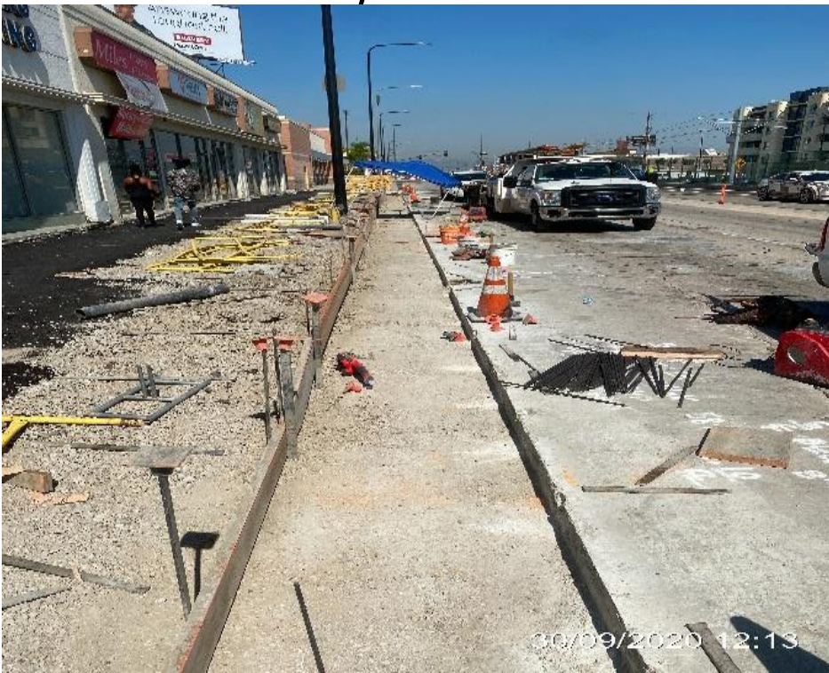
PARK MESA – Placing forms for new curb/gutter installation along SB Crenshaw Blvd between 54th and 57th St.
