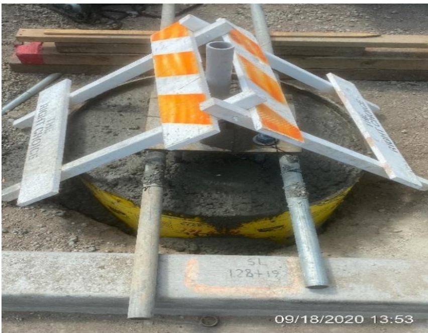
MLK STATION – Placing concrete for street light foundations at the plaza level.
