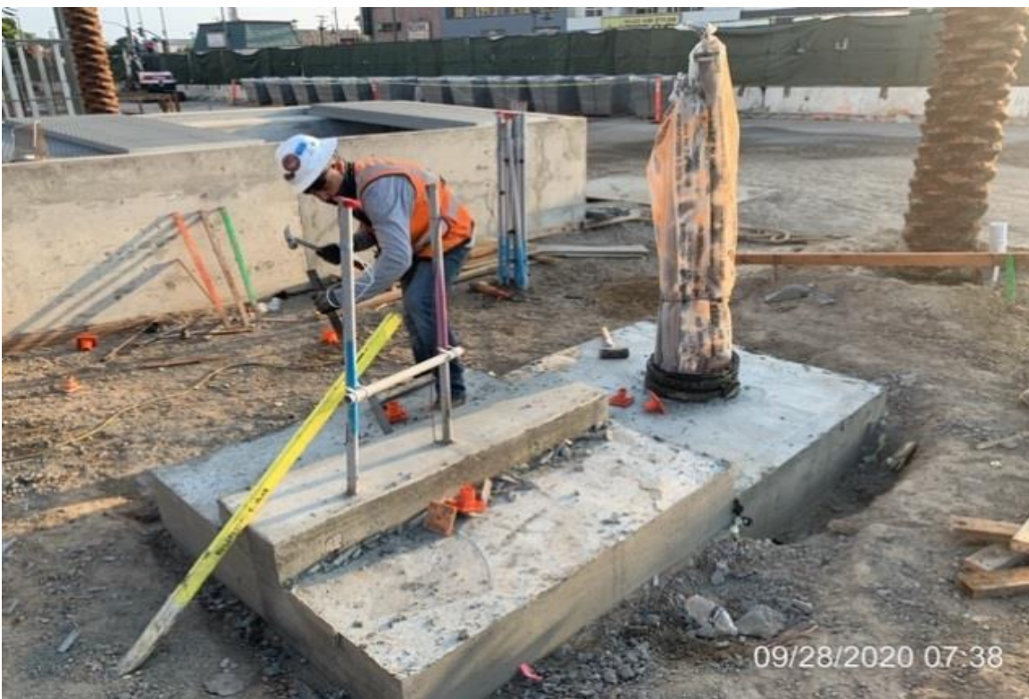
MLK STATION – WSCC carpenters removing formwork from map case and vent stack.
