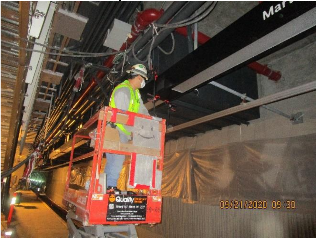
MLK STATION – Continue installing edge light fixtures to the down stand support posts on the north and southbound platform level.
