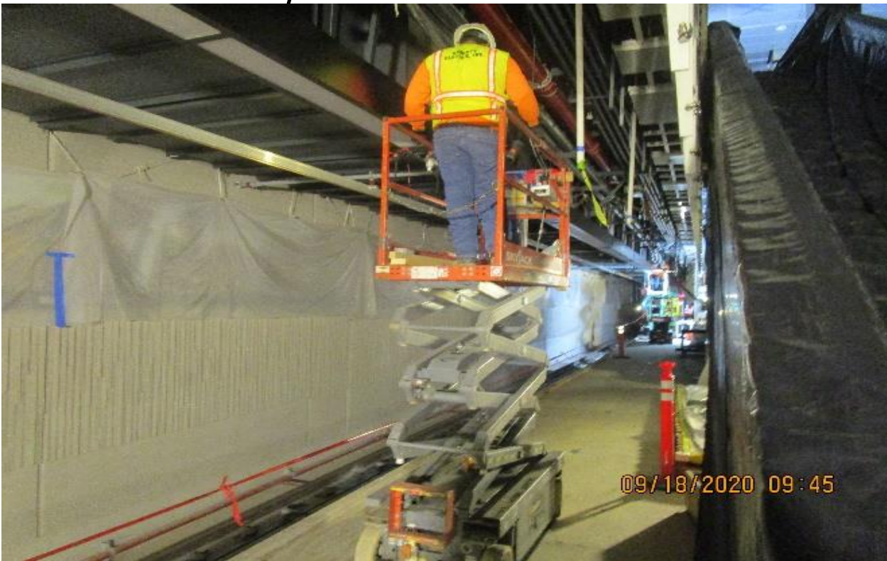
MLK STATION – Continue installing edge light fixtures to the down stand support posts on the southbound platform level..
