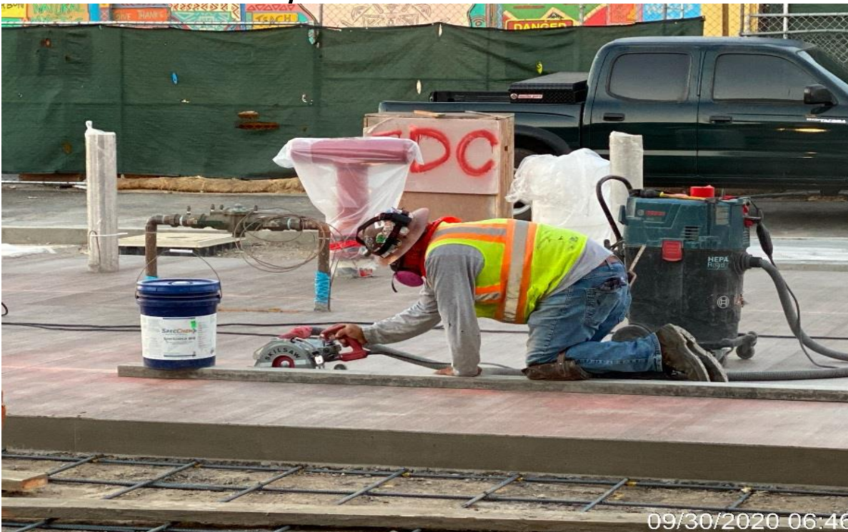
LEIMERT PARK STATION – Continue saw cutting control joints for the architectural topping slab throughout the plaza level.
