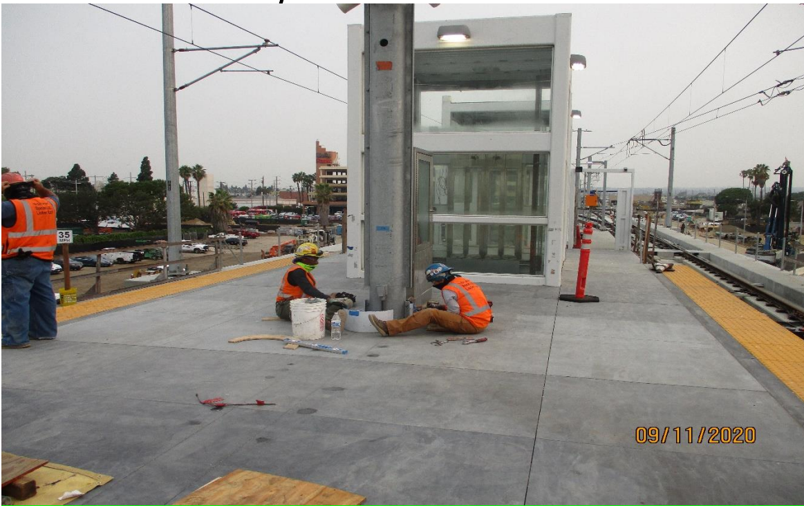
104 th street- Stainless steel cladding being installed at the Aviation Station platform columns.
