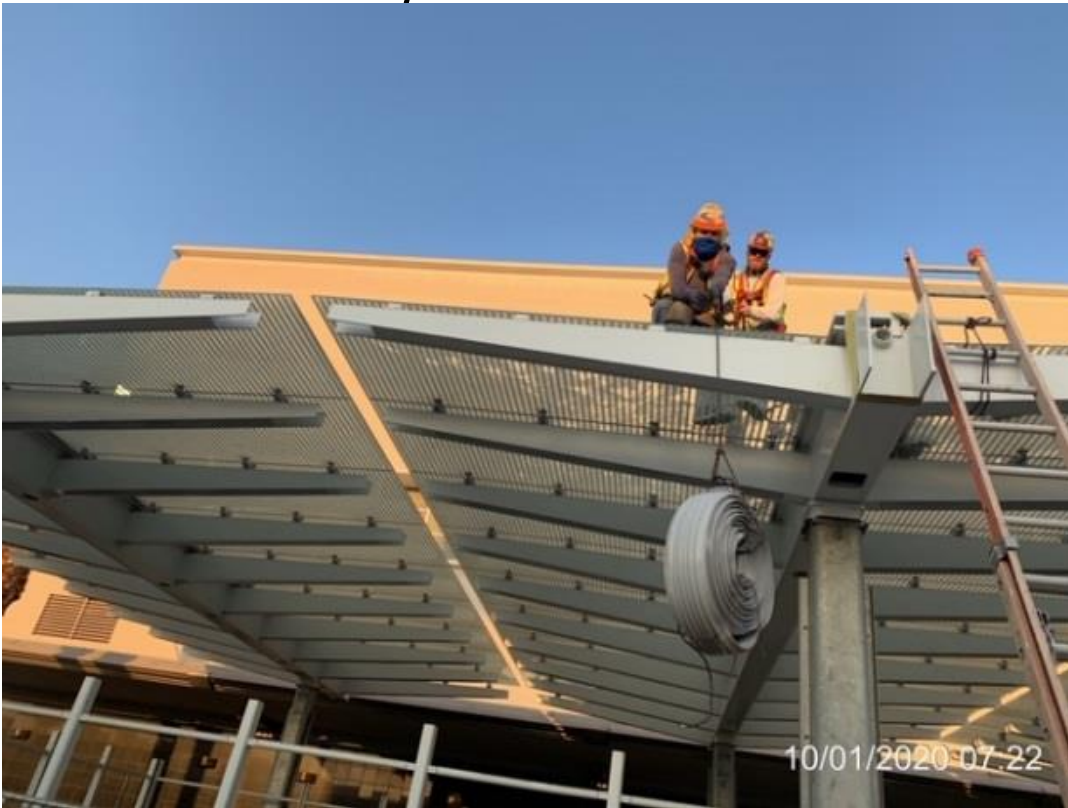
MLK STATION – Caulking and sealing expansion joints for the glass roof of the main entrance canopy at the plaza level.
