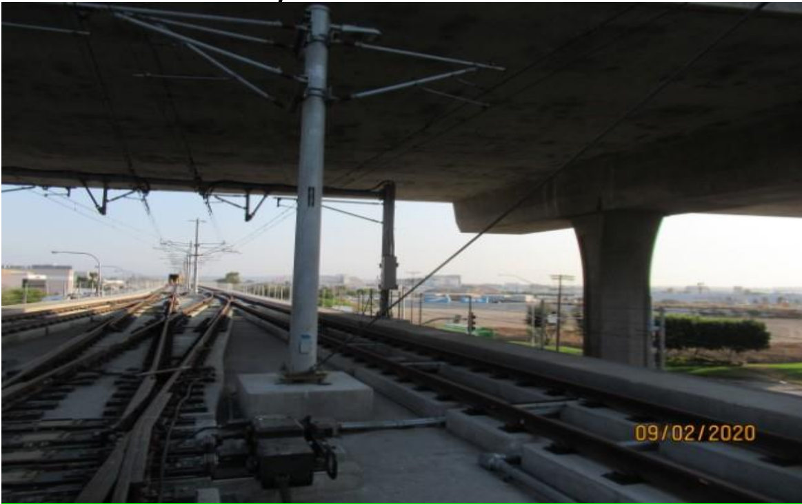
Guideway- OCS pole 1014E at GL Wye Down guy wire still in place over Switch Machine for MPF 3X-ING (looking northeast)
