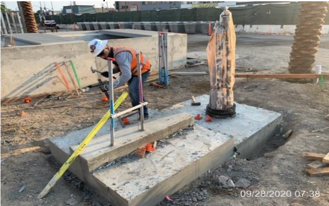
MLK STATION – Removing formwork for the south map case and adjacent plumbing vent stack at the plaza level.
