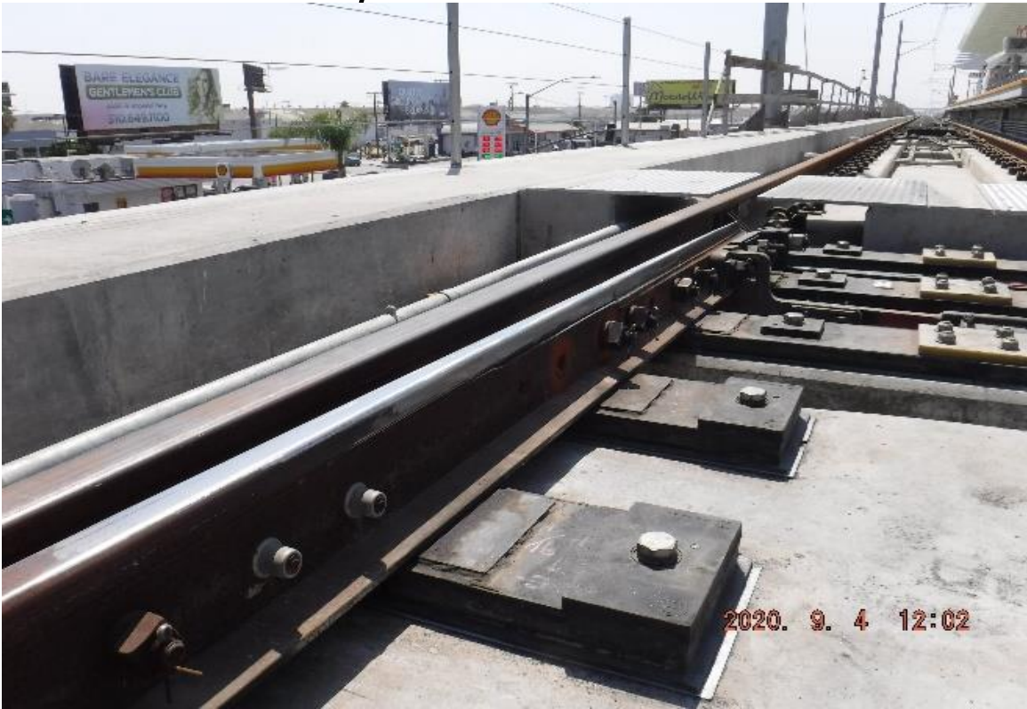
AVIATION/CENTURY- STA 70+11 TK#4/NB looking south – 10K1LHXO switch point manganese insert adjustment (Century)
