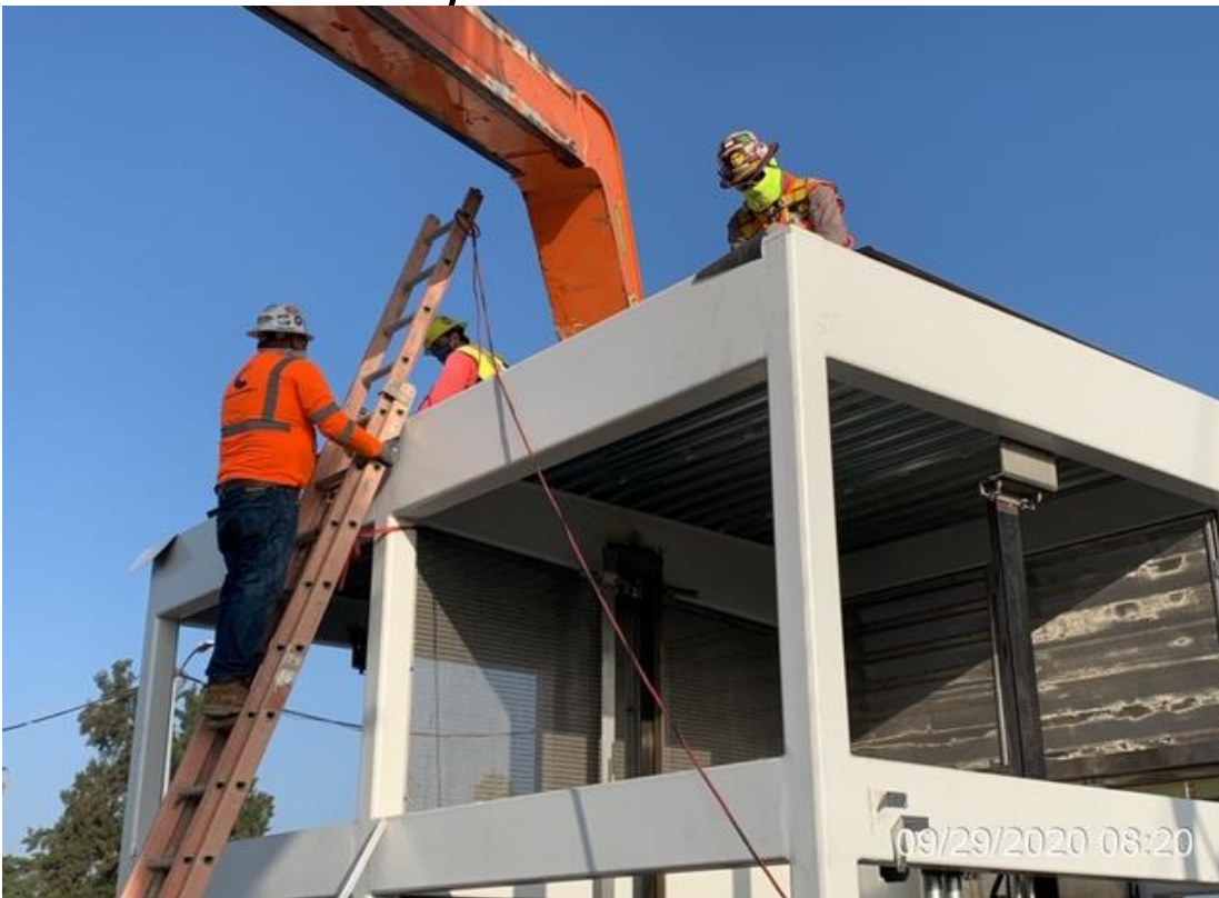
EXPO STATION SITE – Installing membrane and roof decking above Elevators 1&2 at the plaza level.
