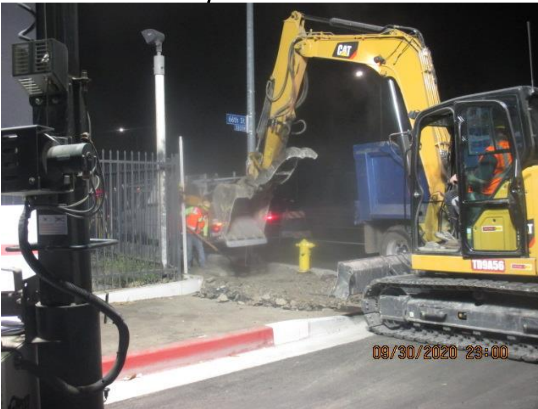
PARK MESA – Excavating/grading for new sidewalk and ADA ramp installation on the northeast corner of 66th St and Crenshaw Blvd.
