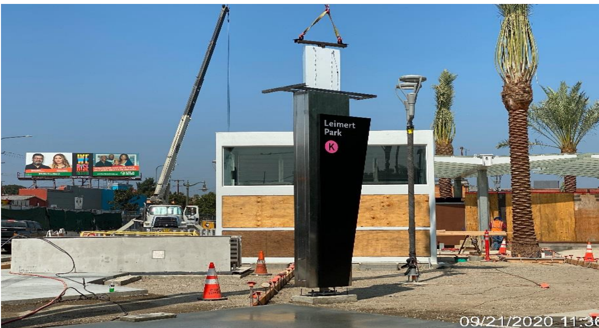
LEIMERT PARK STATION – Installing the Grand Pylon sign at the plaza level.
