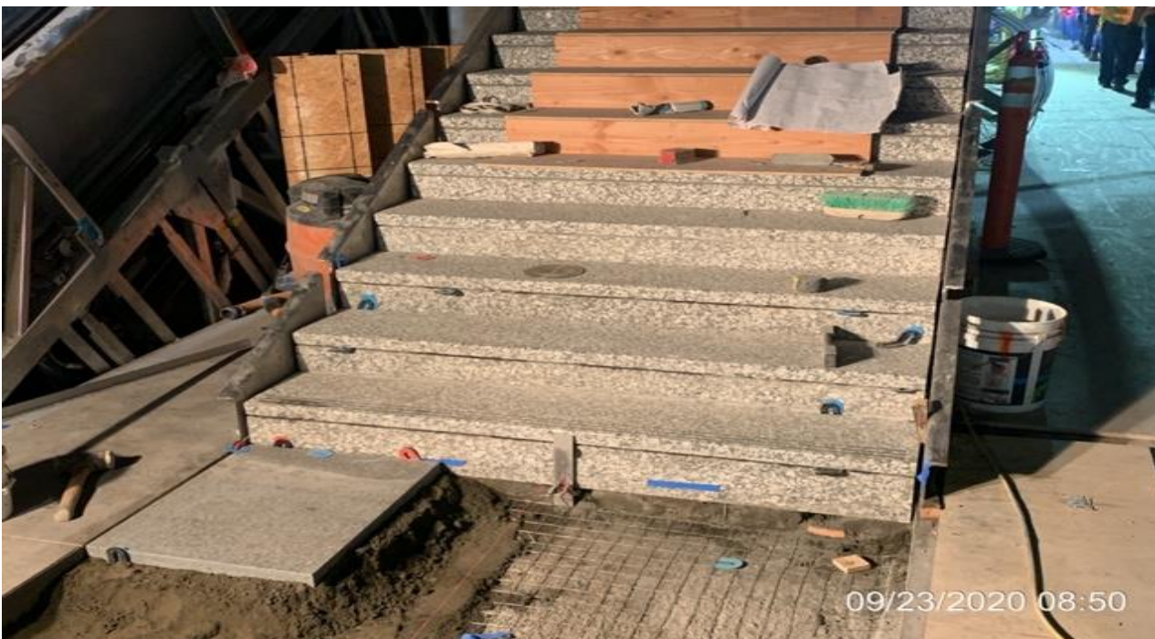
EXPO STATION – Installing granite pavers at the bottom landing of Staircase #2 at the platform level.
