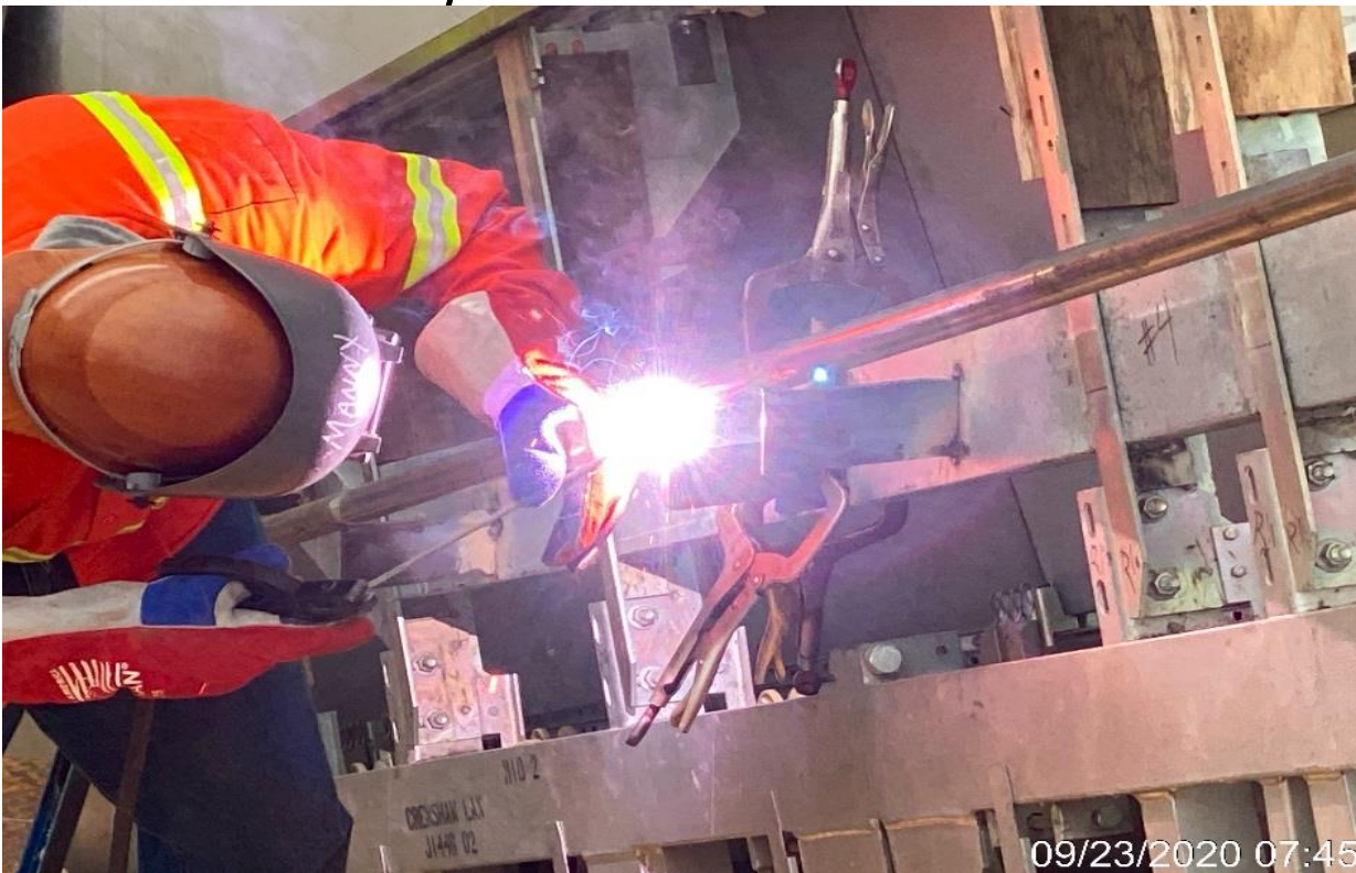
LEIMERT PARK STATION – Continue welding brackets for handrail installation from the intermediate landing to the concourse level.
