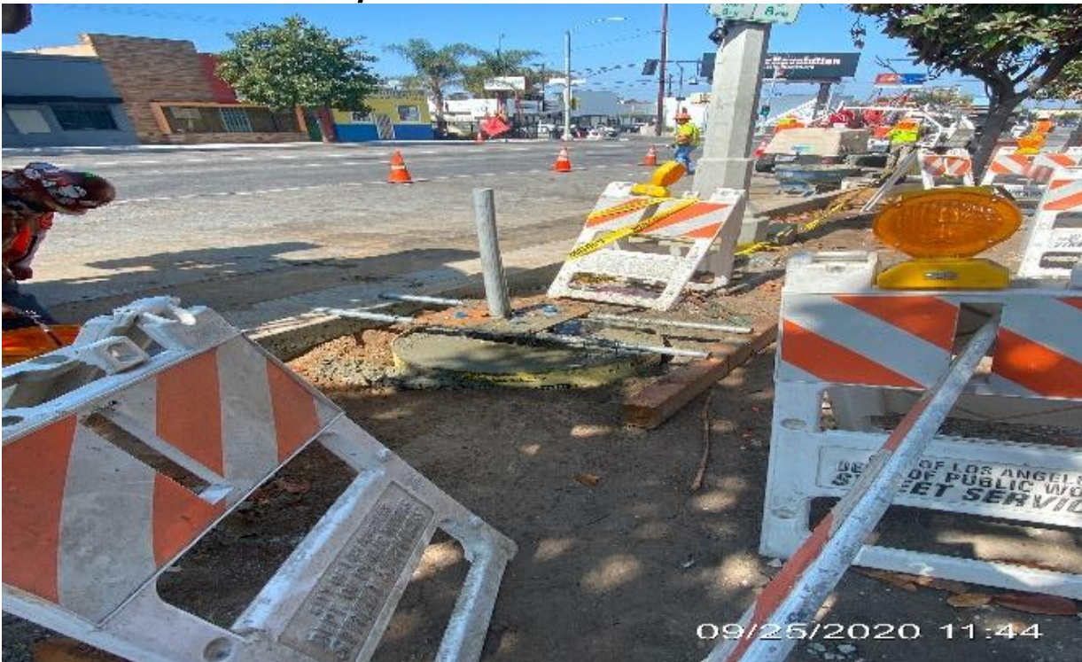
LEIMERT PARK STATION – Placing concrete for pedestrian light poles foundations on Crenshaw Blvd between 43rd Pl and Homeland Dr.
