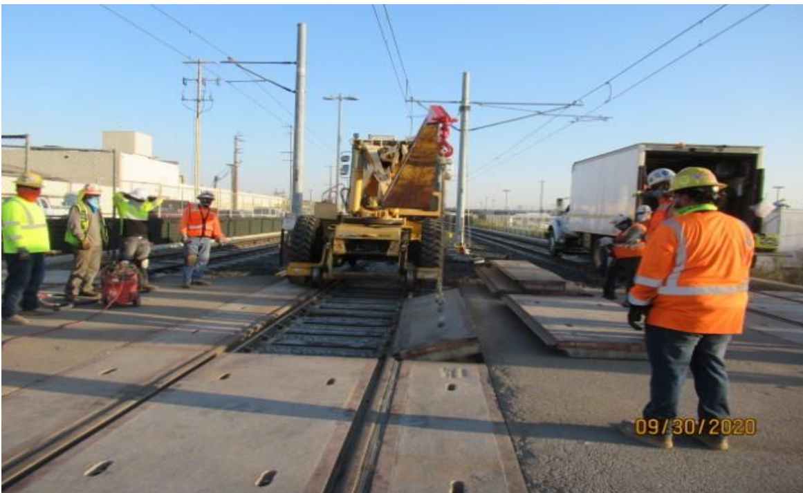
Arbor Vitae- HCC using Speed Swing to remove grade crossing panels at Arbor Vitae for damaged rail replacement (looking north) Rework
