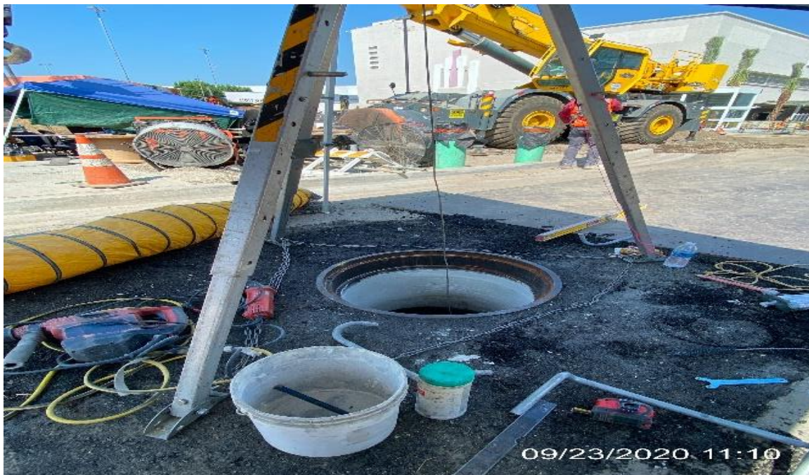
MLK STATION – Preparing Manholes #10 and #16 for pre-final inspections along the plaza level.
