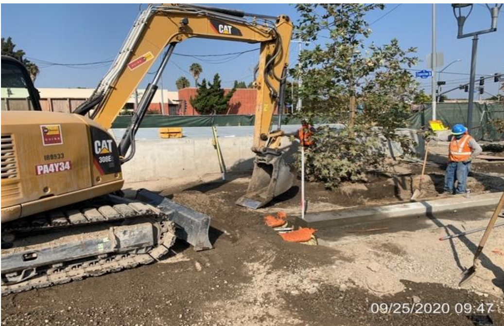
EXPO STATION – Continue backfilling/grading the north end area of the plaza level.
