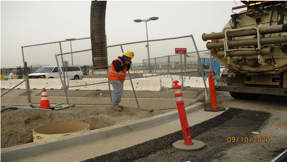
104 th street- Vacuum truck excavating for a traffic signal pole at Aviation and 104th.
