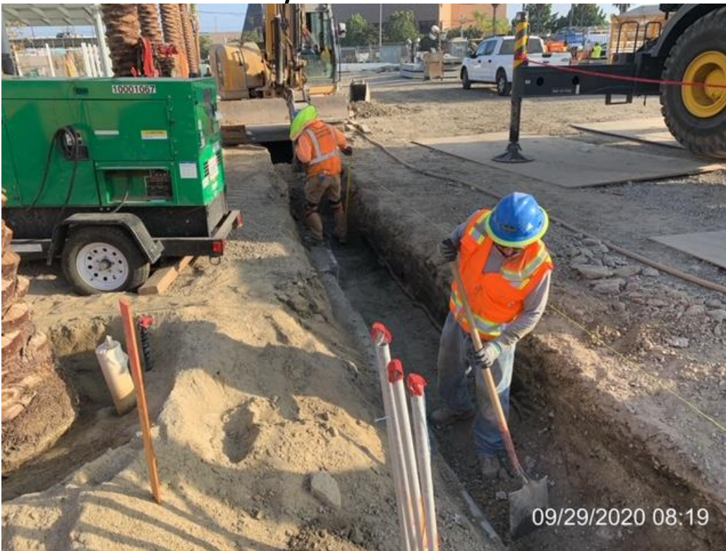
EXPO STATION – Continue excavating for the east side bollard foundations at the plaza level.
