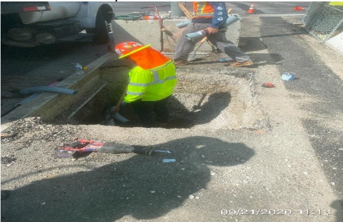
EXPO STATION - Continue installing AT&T conduit and preparing for vault installation on the northeast corner of Obama Blvd and Crenshaw Blvd.
