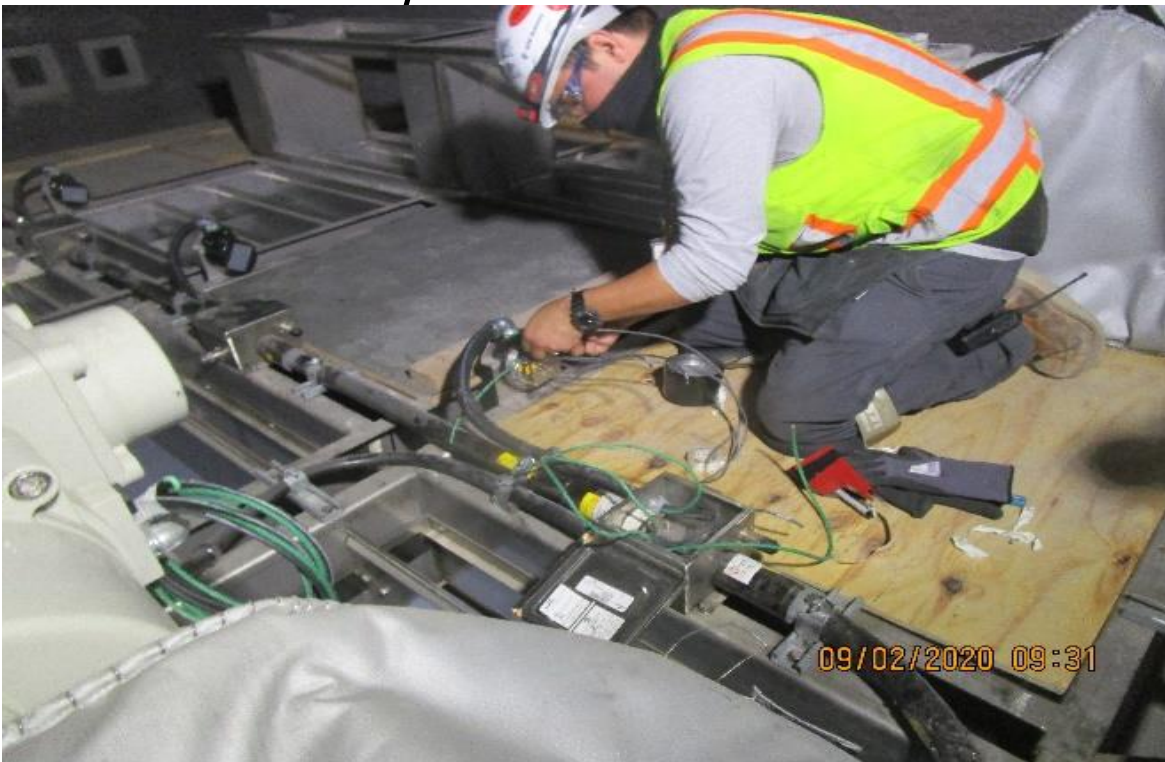
MLK STATION – Tunnel vent plenum OTE (S) C101, TD-7-121, begin identify, label, & dress limit switch load conductors.
