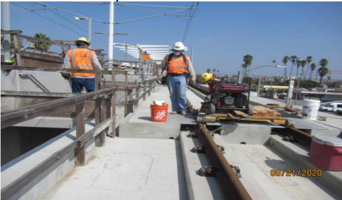
AVIATION/CENTURY- Century/Aviation Bridge NB track STA 66+28 WSCC repair work on Emergency Walkway Crossing plates (looking north)
