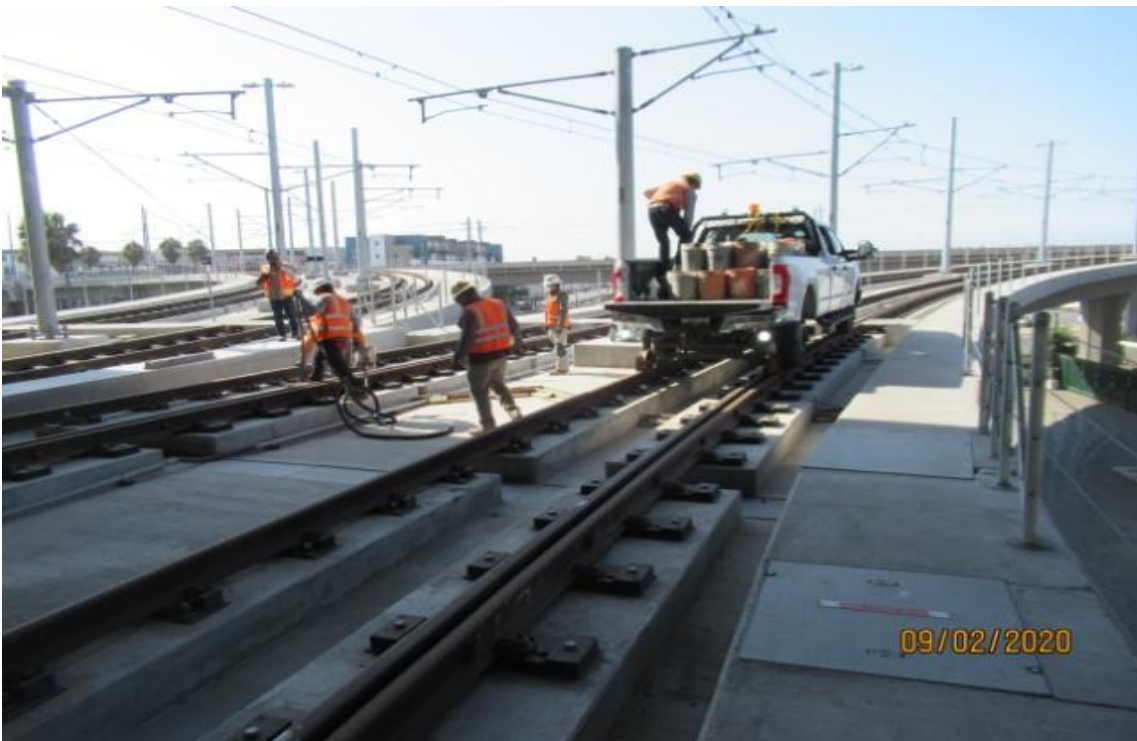
Guideway- WSCC Concrete repair crew on west leg of Wye placing concrete for plinth repair work (looking south) Rework for NCR-A 111-B case 4
