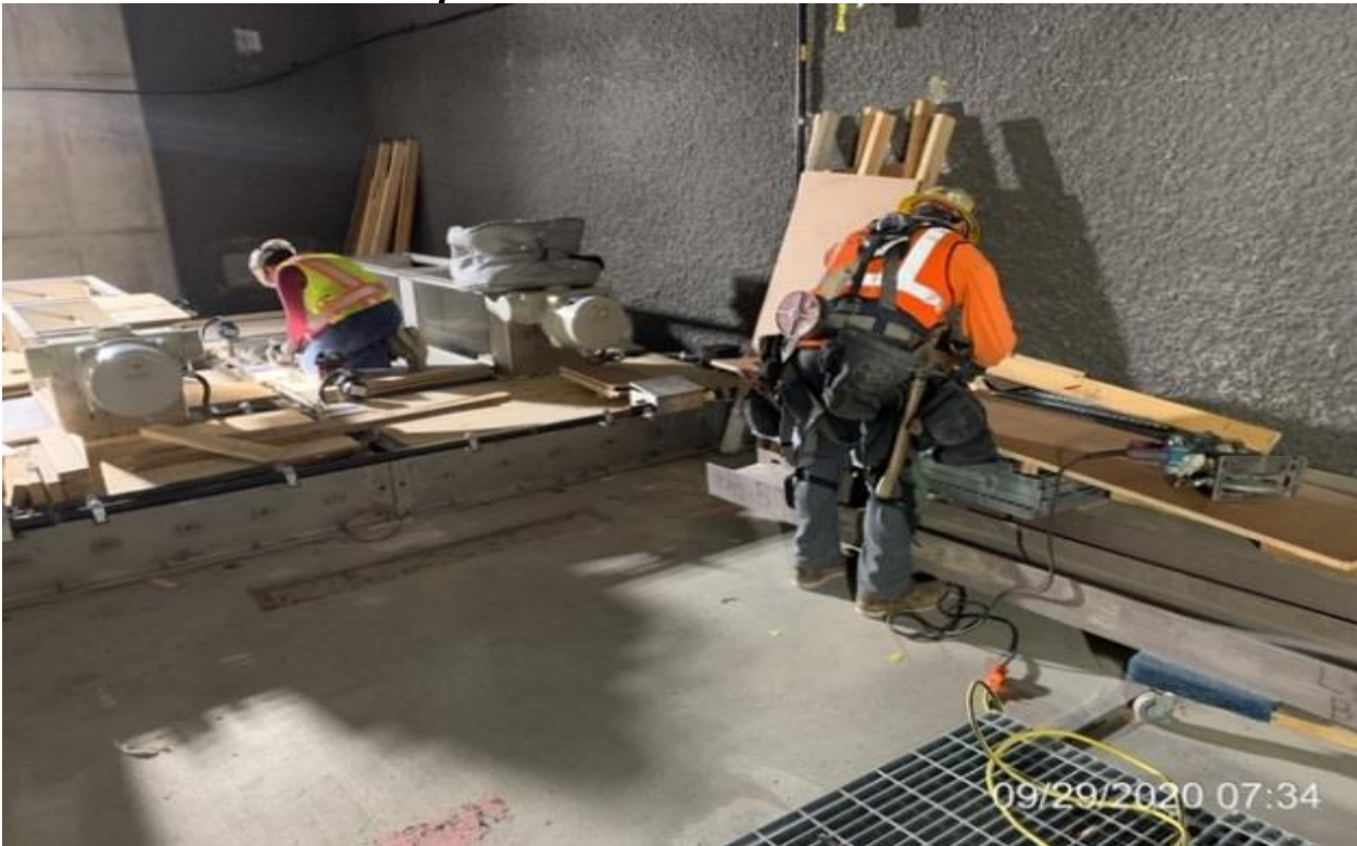
MLK STATION – Continue building formwork for catwalk pedestal bases inside the South EVF Room at the concourse level.
