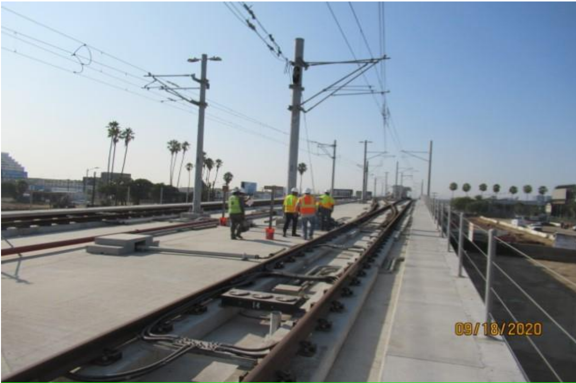
AVIATION/CENTURY- Century/Aviation Bridge 10K2LHXO SB track POS STA 73+96 Metro Operations & LKC personal on site for Switch Point ¼" Obstruction (looking south)
