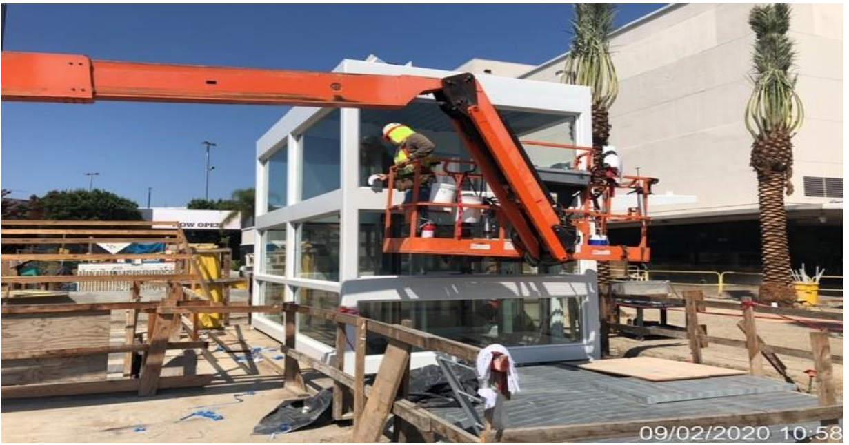
MLK STATION – Giroux Glass applying caulking to glass panels for elevator structure #1 and #2
