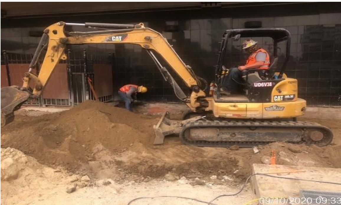
MLK STATION – WSCC crew excavating to grade along foundation of mall Bldg. for new walkway..
