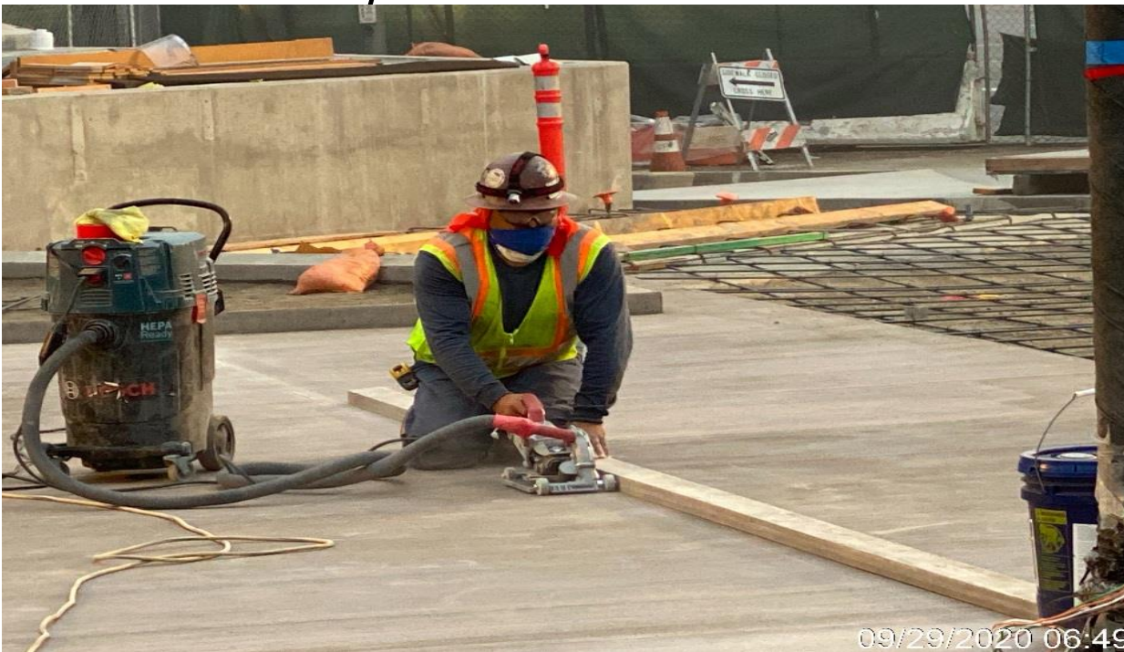
LEIMERT PARK STATION – Saw cutting control joints for the architectural topping slab throughout the plaza level.
