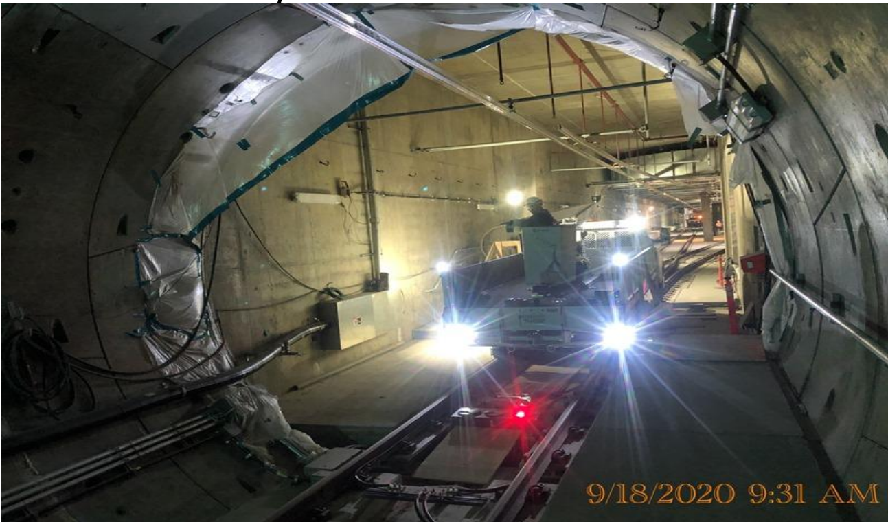
EXPO STATION – Continue installing supports and fixtures for the crossover lighting at the invert level.
