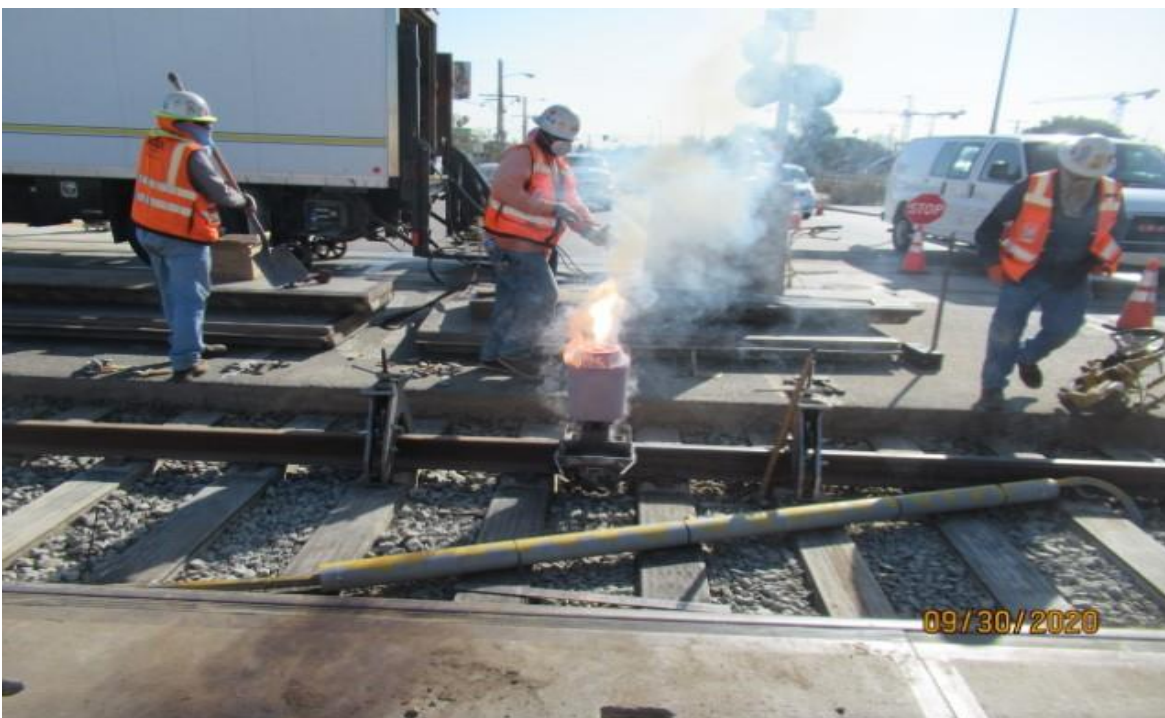
Arbor Vitae- LKC removing system loop O-bonds inside Arbor Vitae grade crossing SB track between STA 93+77 & 94+33 (looking south) Rework RFI-01499
