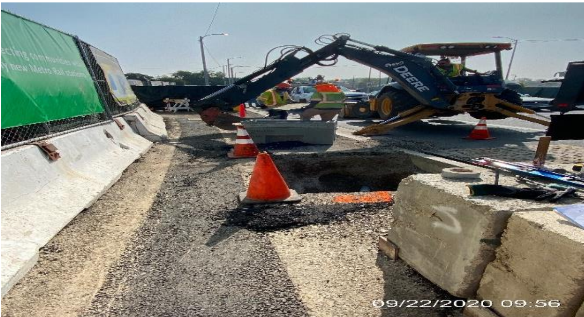
EXPO STATION – Continue installing AT&T conduit and setting fiber vault on the northeast corner of Obama Blvd and Crenshaw Blvd.
