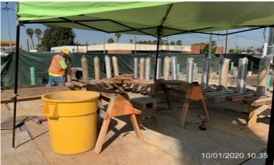
EXPO STATION – Preparing to install the bollard on the east side trench of the plaza level.
