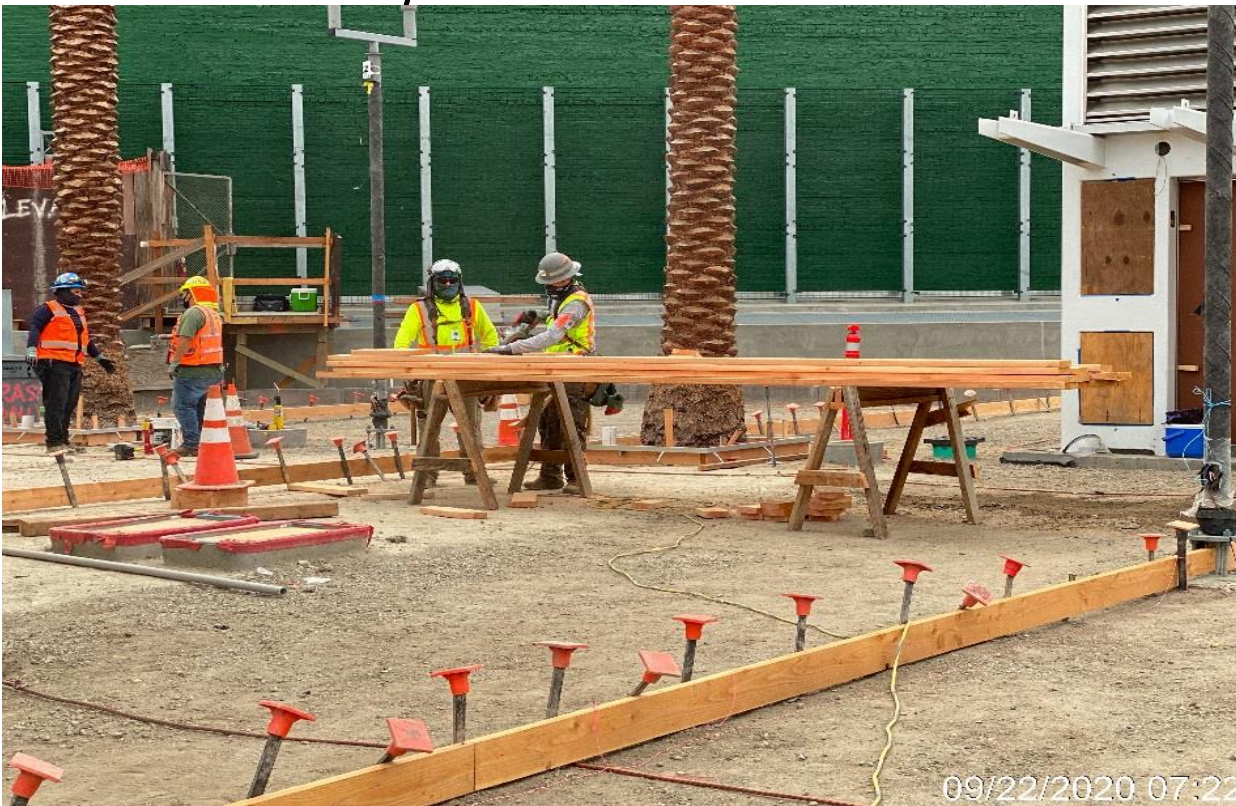
LEIMERT PARK STATION – Continue setting forms for concrete placement of the architectural topping slab throughout the plaza level.
