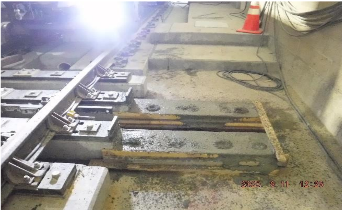
UG4 – STA 440+65 TK#4,NB looking south – 8W1 switch machine plinth pour – UG4 Expo DXO
