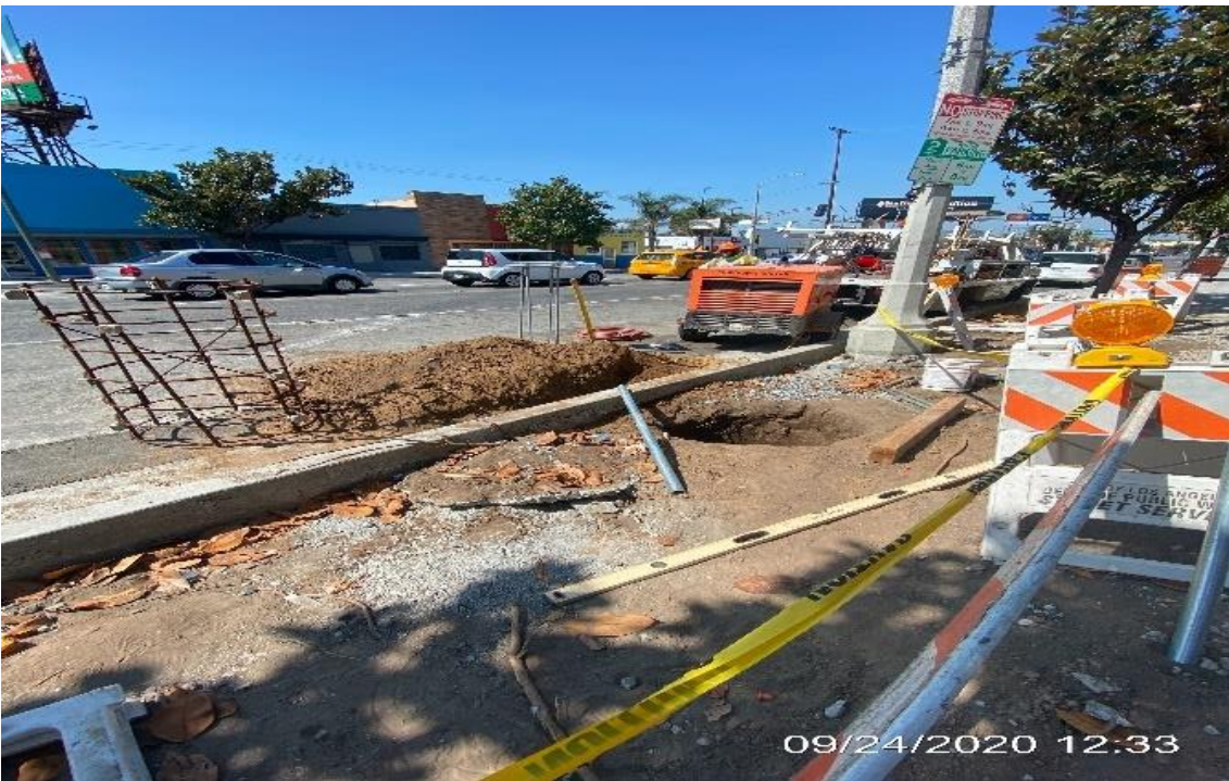
LEIMERT PARK STATION – Preparing to set rebar and foundations for pedestrian light poles on Crenshaw Blvd between 43rd Pl and Homeland Dr.
