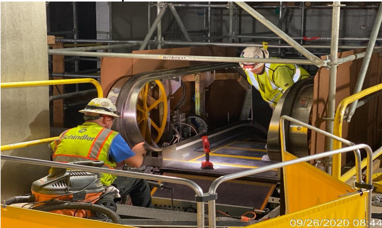
EXPO STATION – Performing start-up and energization work for all Escalators 3&4 at the concourse level.
