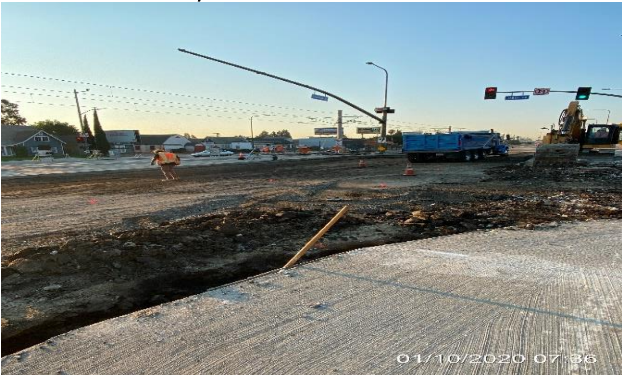
PARK MESA – Continue excavating and backfilling the roadway intersection on Crenshaw Blvd and 48th St.
