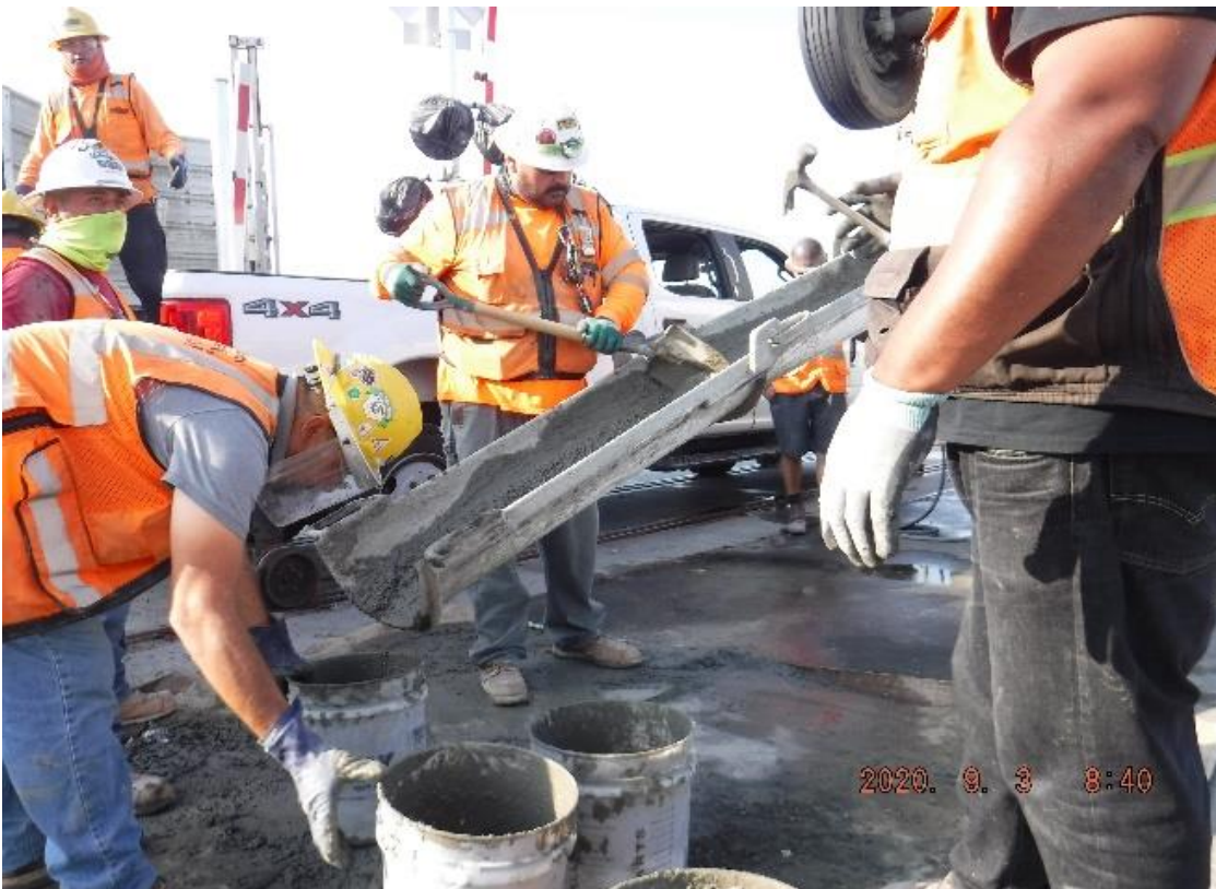
UG3 – STA 273+30 TK#4/NB looking east – unloading PCC for NCR-A-111.B Case #4 work in UG3 (Brynhurst)
