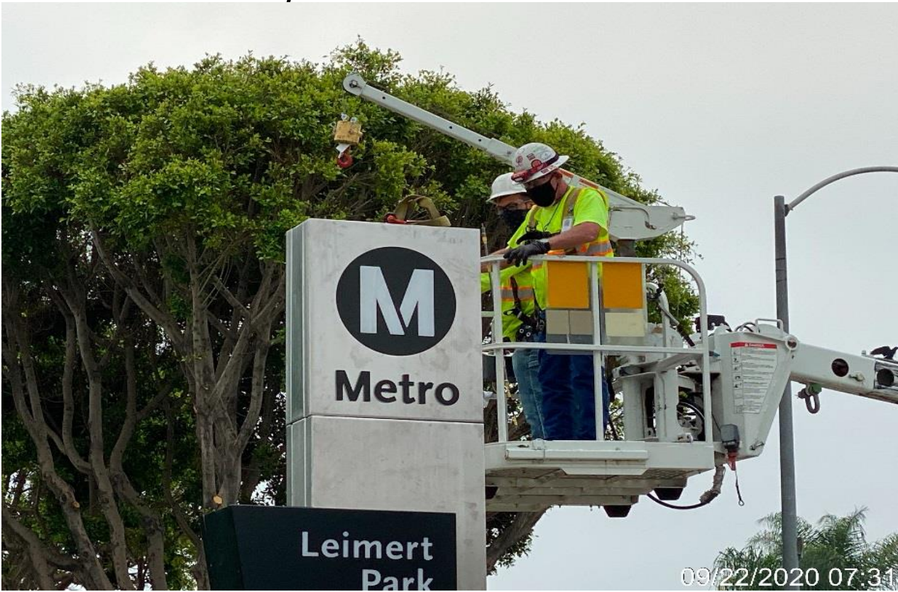
LEIMERT PARK STATION – Continue installing the Grand Pylon sign at the plaza level.
