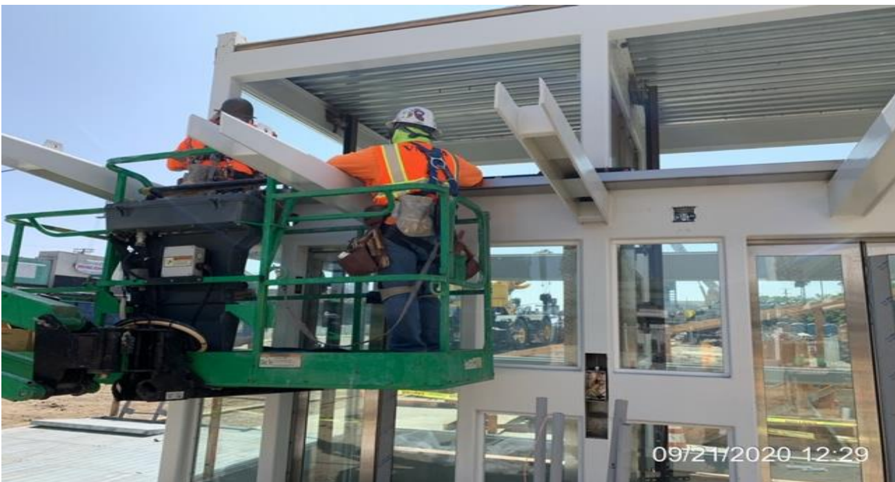
MLK STATION – Installing louvers and gutters to Elevators 1&2 at the plaza level.
