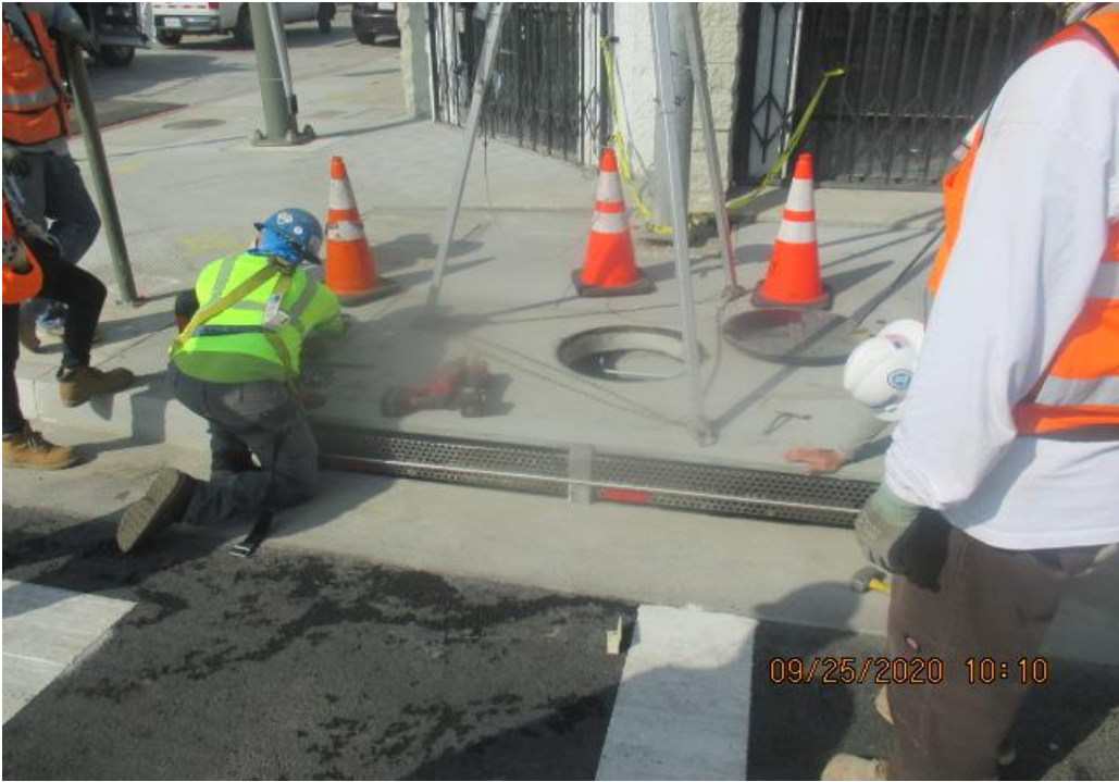
PARK MESA – Installed grate for Catch Basin #30 and #31 on the northwest corner of Crenshaw Blvd and 67th St.
