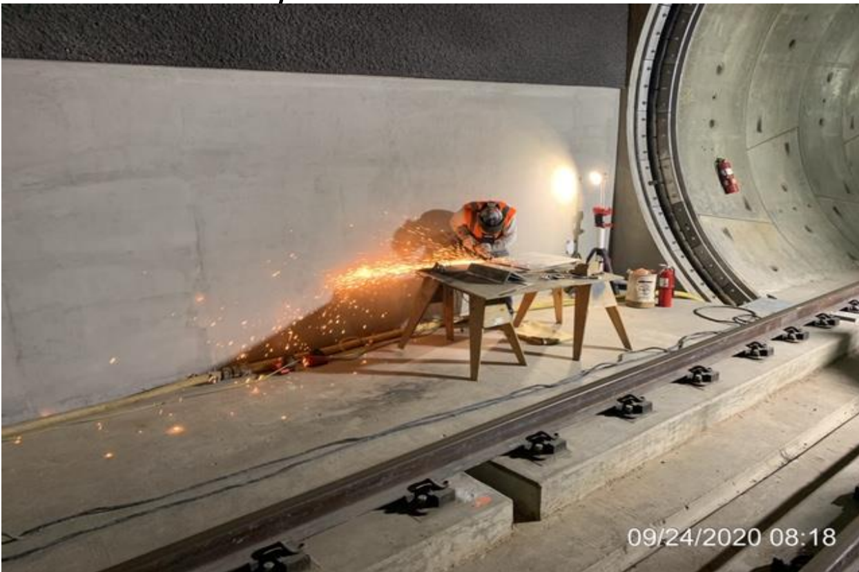
MLK STATION – Installing crossover plates along the North Back of House emergency walkway at the northbound platform level.
