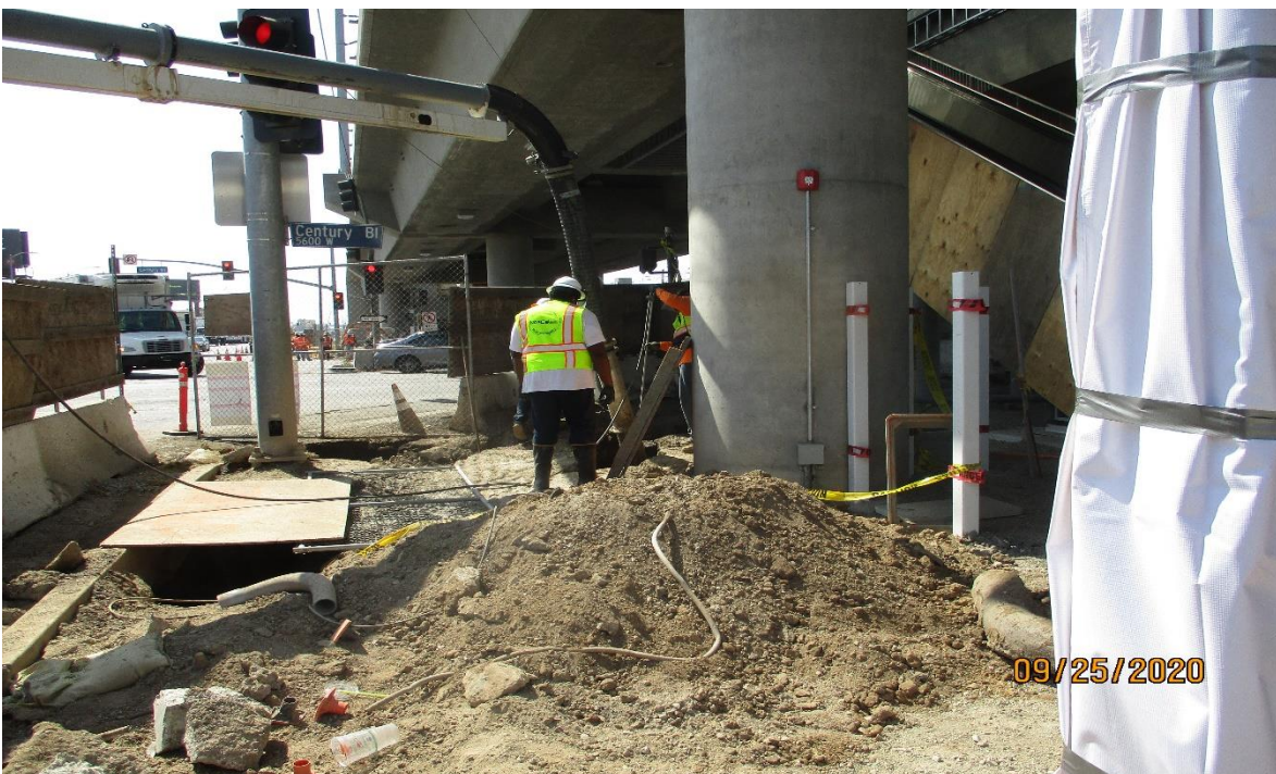
AVIATION/CENTURY- Daylighting obstructions for the traffic signal conduit on the NW corner of Aviation and Century.
