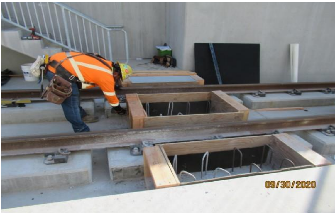
UG1- WSCC carpenter adjusting concrete foundation forms for Emergency Walkway Crossings at UG1 NB track STA 56+50 Rework
