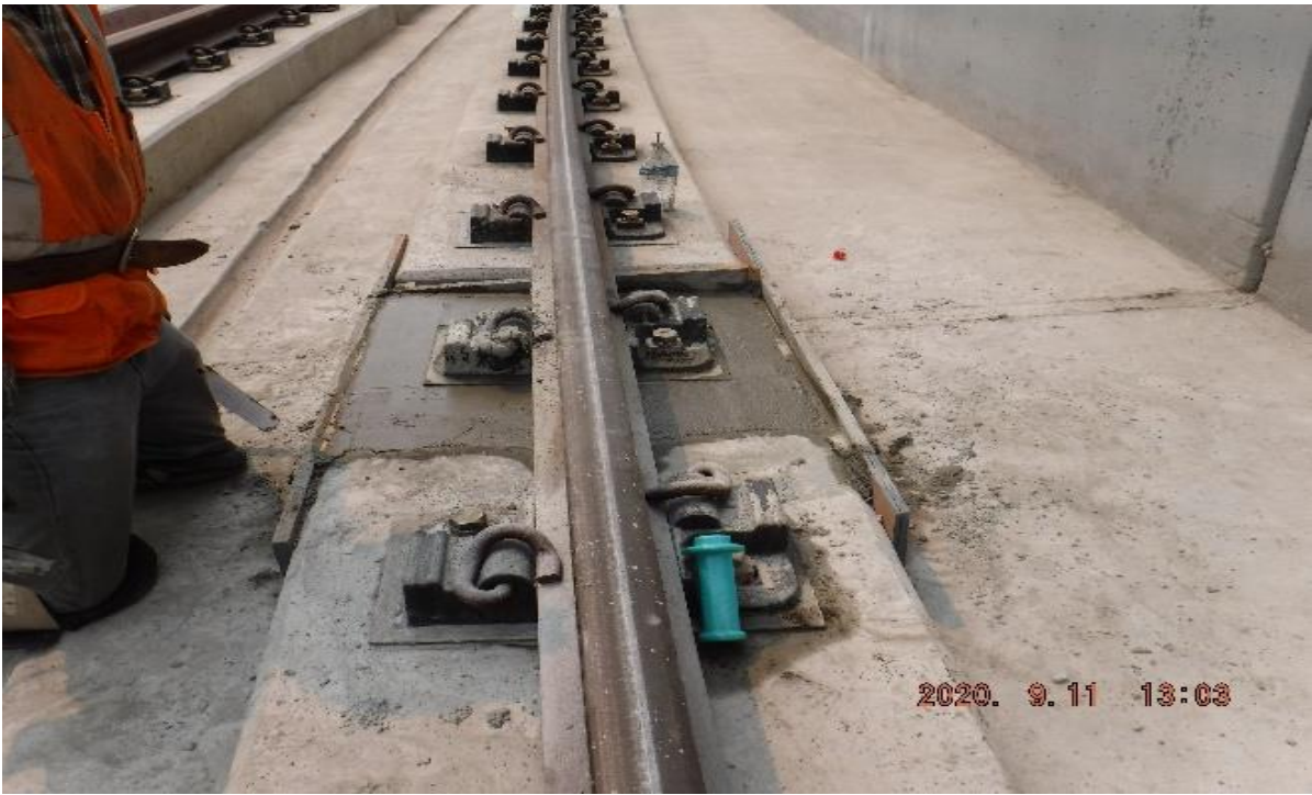
UG3 – STA 281+48 TK#3/SB looking south – NCR-A-111.B – left plinth DF #287 fresh PCC top surface finishing in prog104ress – UG3
