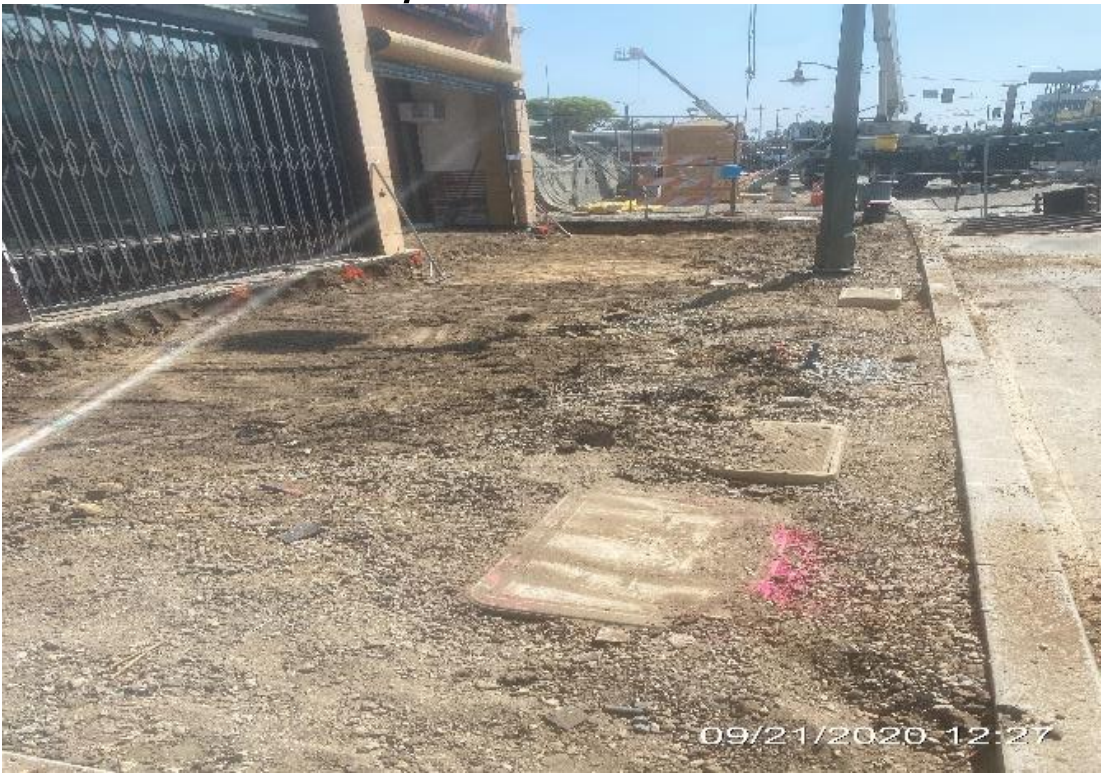
LEIMERT PARK STATION SITE – Excavating portion of sidewalk panels for restoration on northbound Crenshaw Blvd near the far northwest corner of the plaza.
