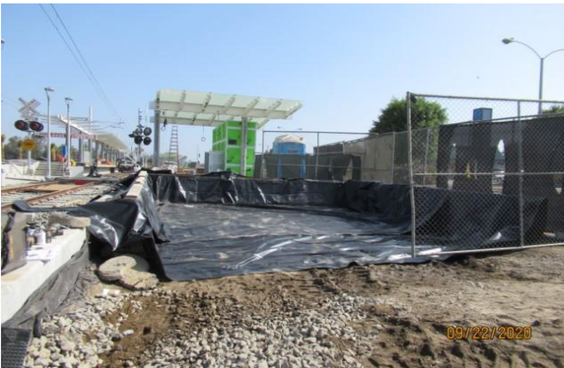
La Brea – La Brea wall 202 off NB track at approximate STA 208+25 WSCC assembling pit for Vacuum truck dump area Rework NCR B-089
