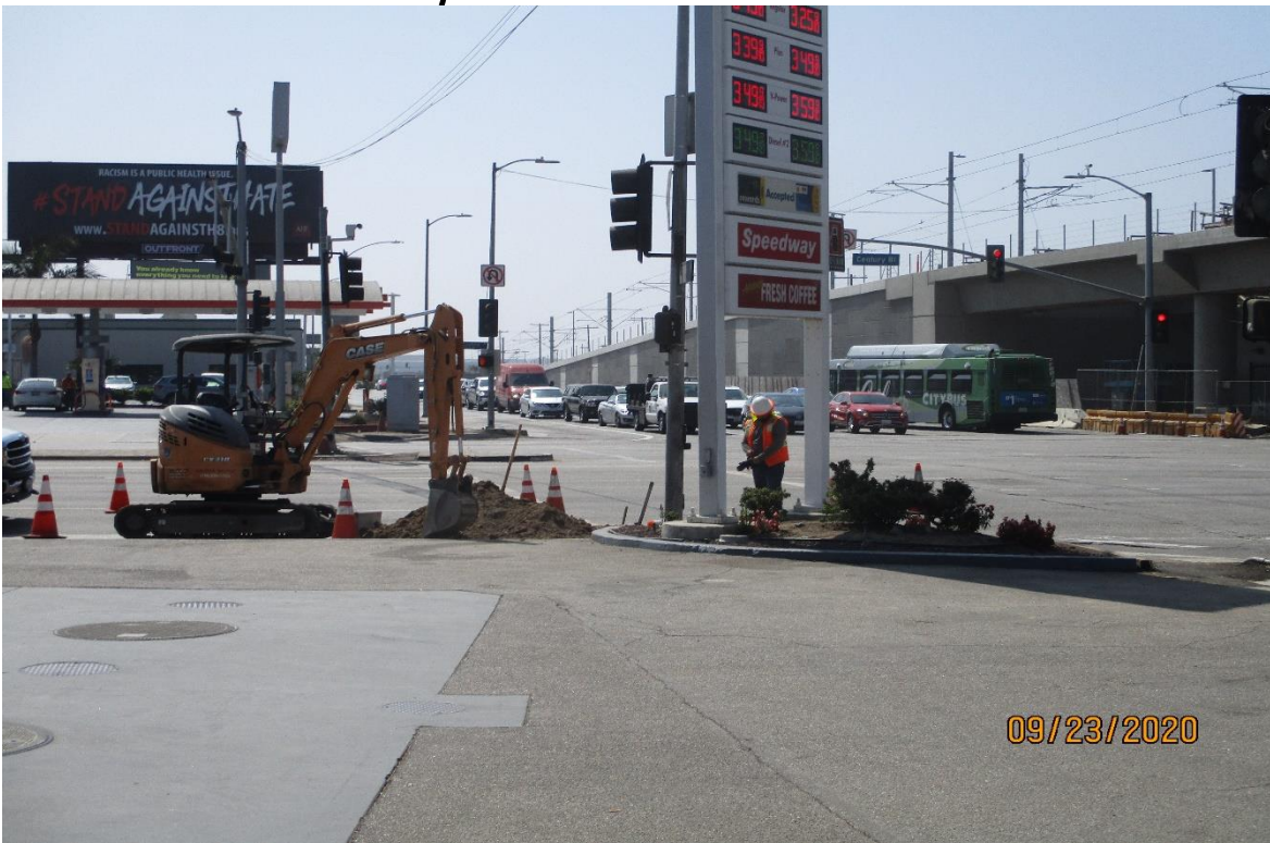
AVIATION/CENTURY- Traffic signal conduit work at the intersection of Aviation and Century.
