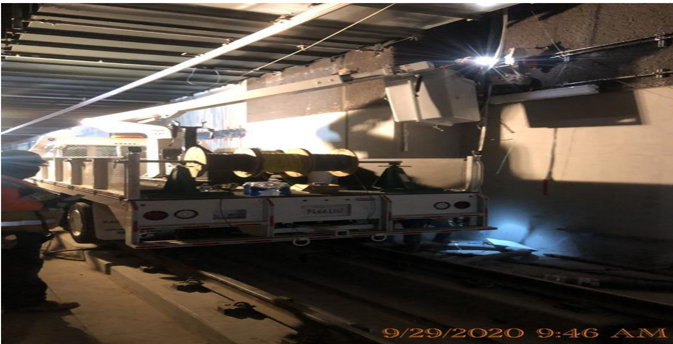
EXPO STATION – Continue installing supports and fixtures for the crossover lighting at the invert level.
