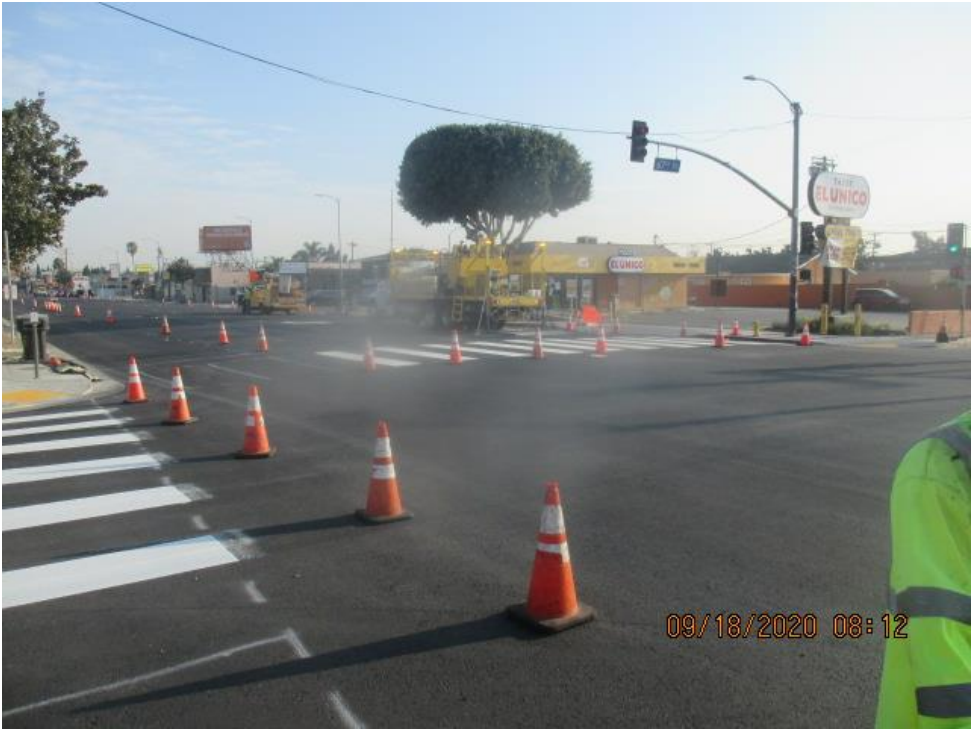
Park Mesa – Lane striping and painting pedestrian crossings on north and southbound Crenshaw Blvd from 67th St to 60th St.
