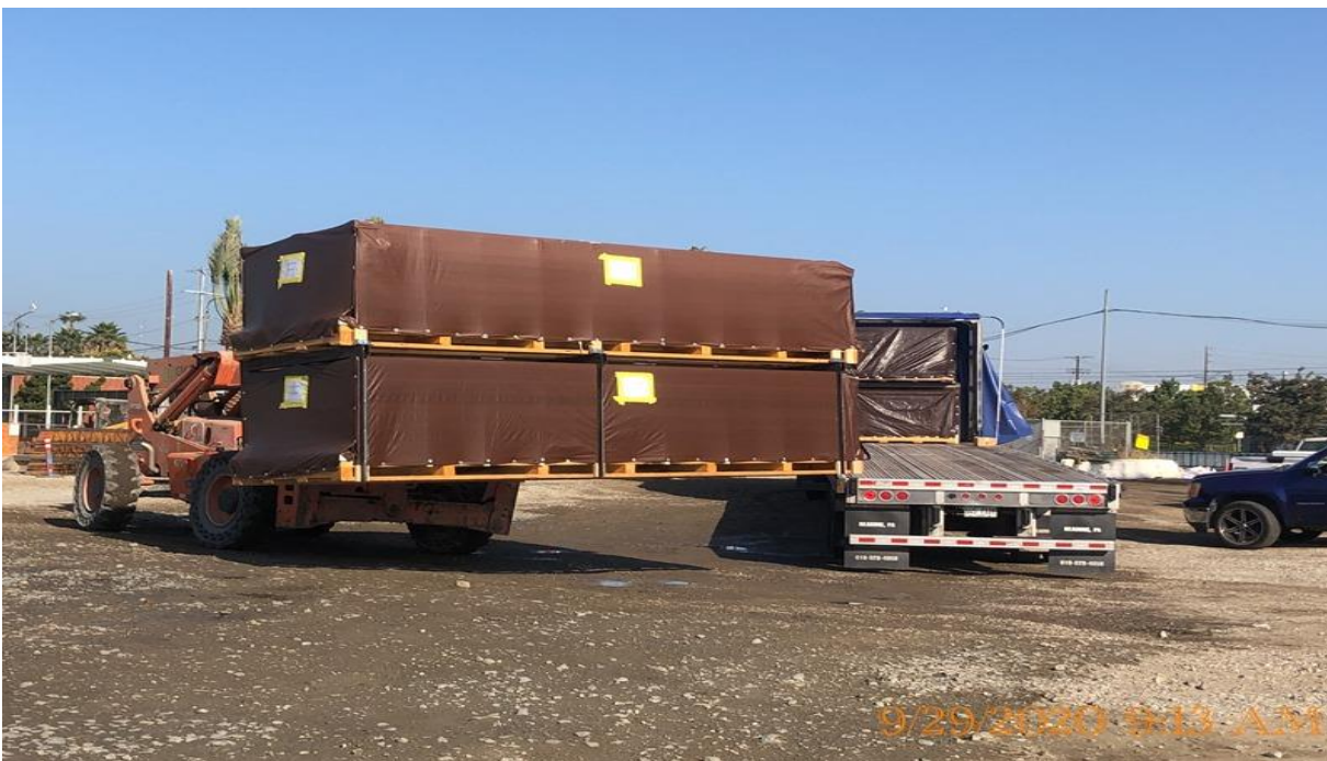
EXPO STATION SITE – Delivering the platform edge lights at the plaza level.
