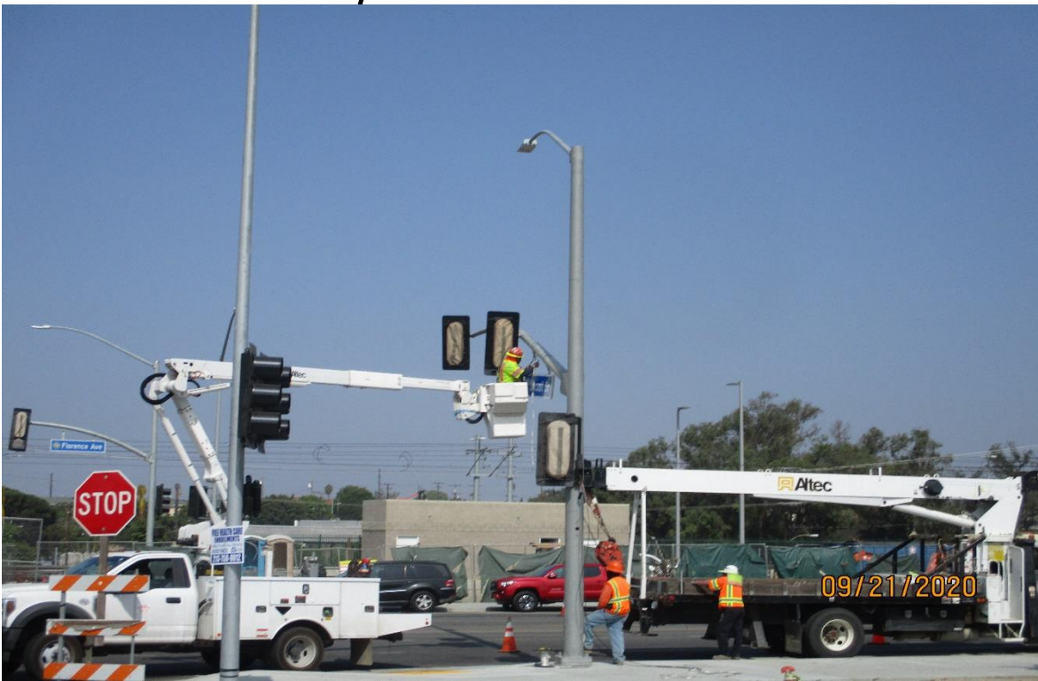
Hindry – Installing the street sign on the mast arm at Locust and Florence.
