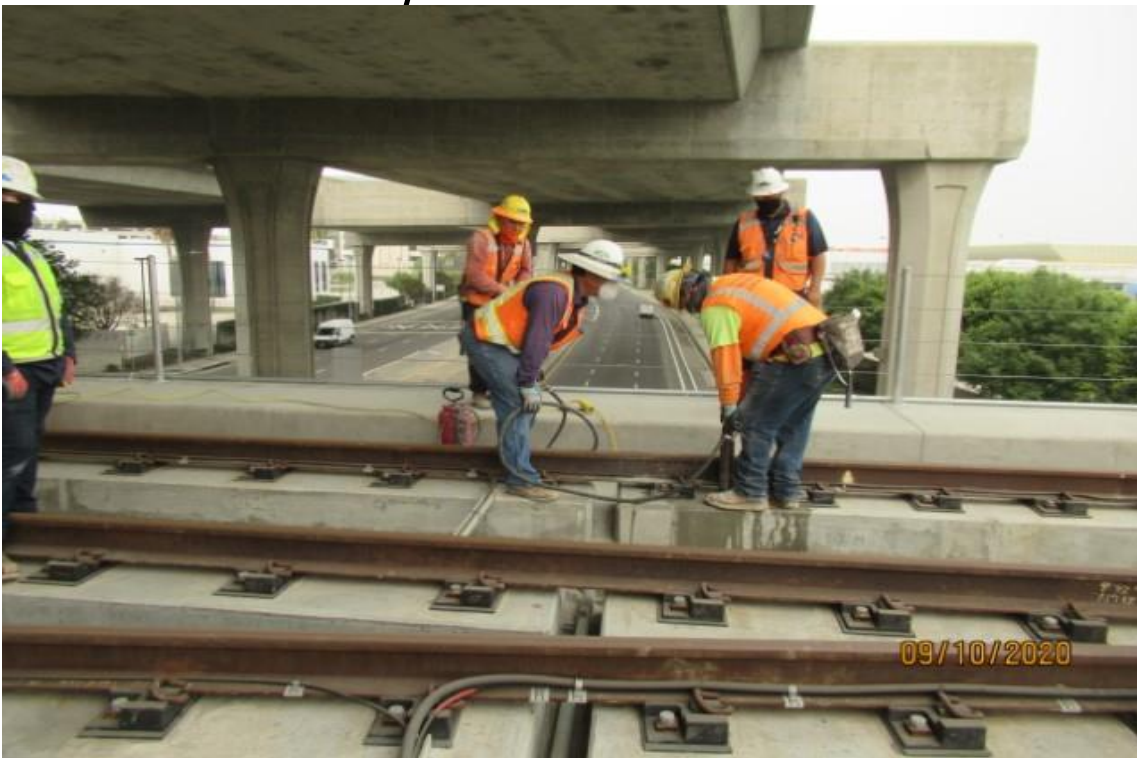
Guideway- WSCC on SBW track at GL Wye left side plinth core drilling concrete sample for re-testing break strength (looking west) Rework
