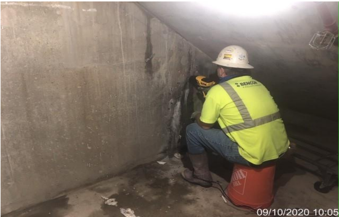
MLK STATION – Keller injecting polyurethane sealant to mediate water intrusion at emergency exit stair #2
