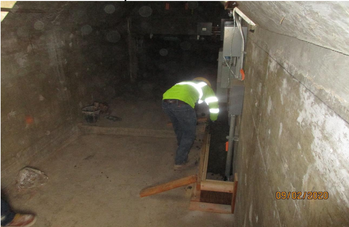
Hindry – Placing concrete to encase some electrical conduit in the west end of the SB Hindry Station platform.
