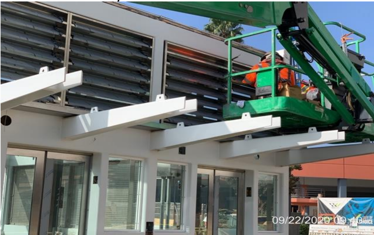
MLK STATION – Continue installing louvers and gutters to Elevators 1&2 at the plaza level.
