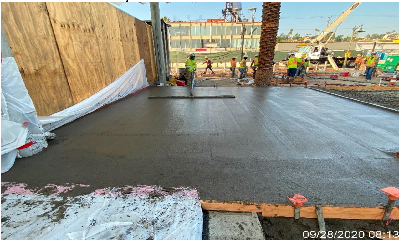
LEIMERT PARK STATION – Placing concrete for the architectural topping slab throughout the plaza level.
