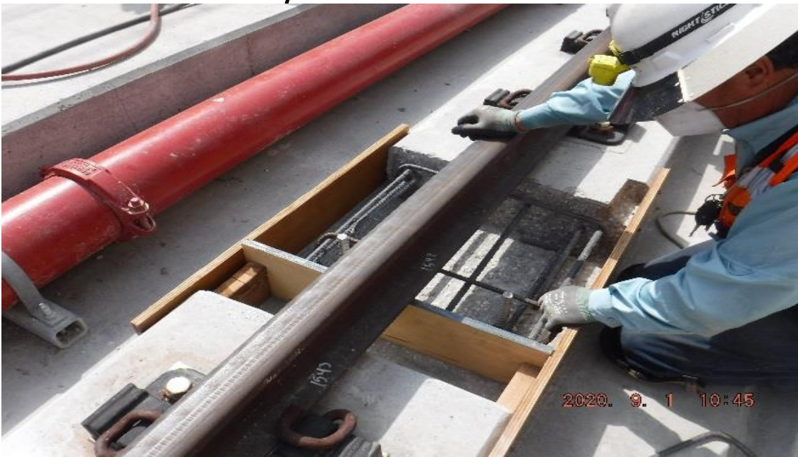
UG3 – STA 312+95 TK#3/SB looking south – dowels epoxy set-up part of NCR-A-111.B Case #4 UG3 (Victoria)
