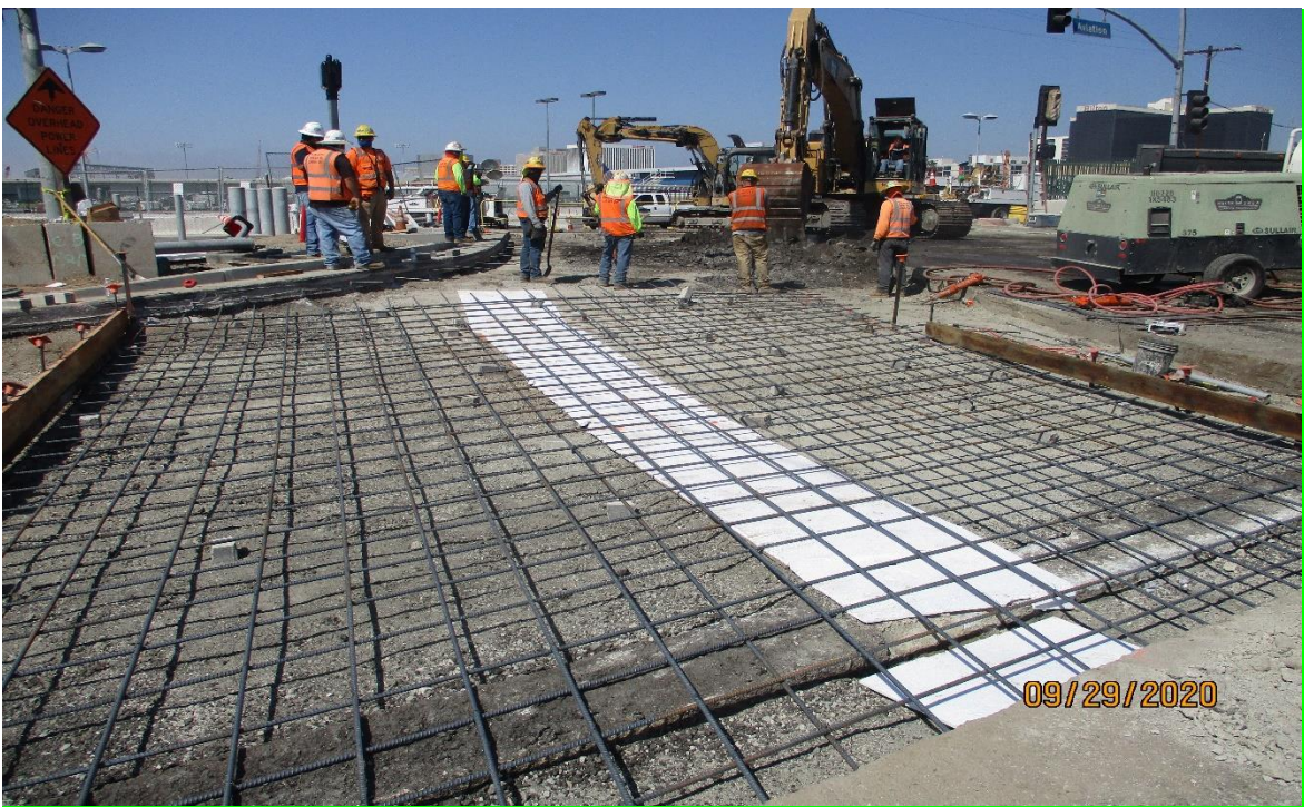
104 th street- Start of the placement of the rebar for the protection slab at 104th street.
