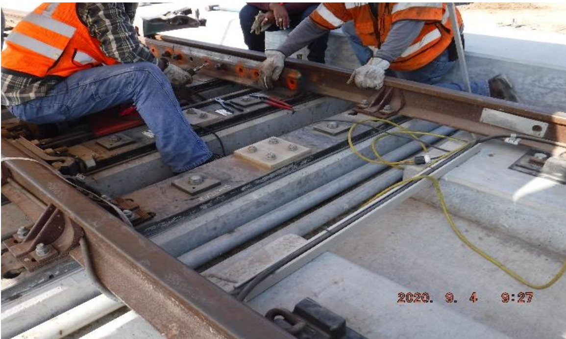
AVIATION/CENTURY- STA 73+95 TK#3/SB looking west – 10K2LHXO switch point manganese insert adjustment (Century)
