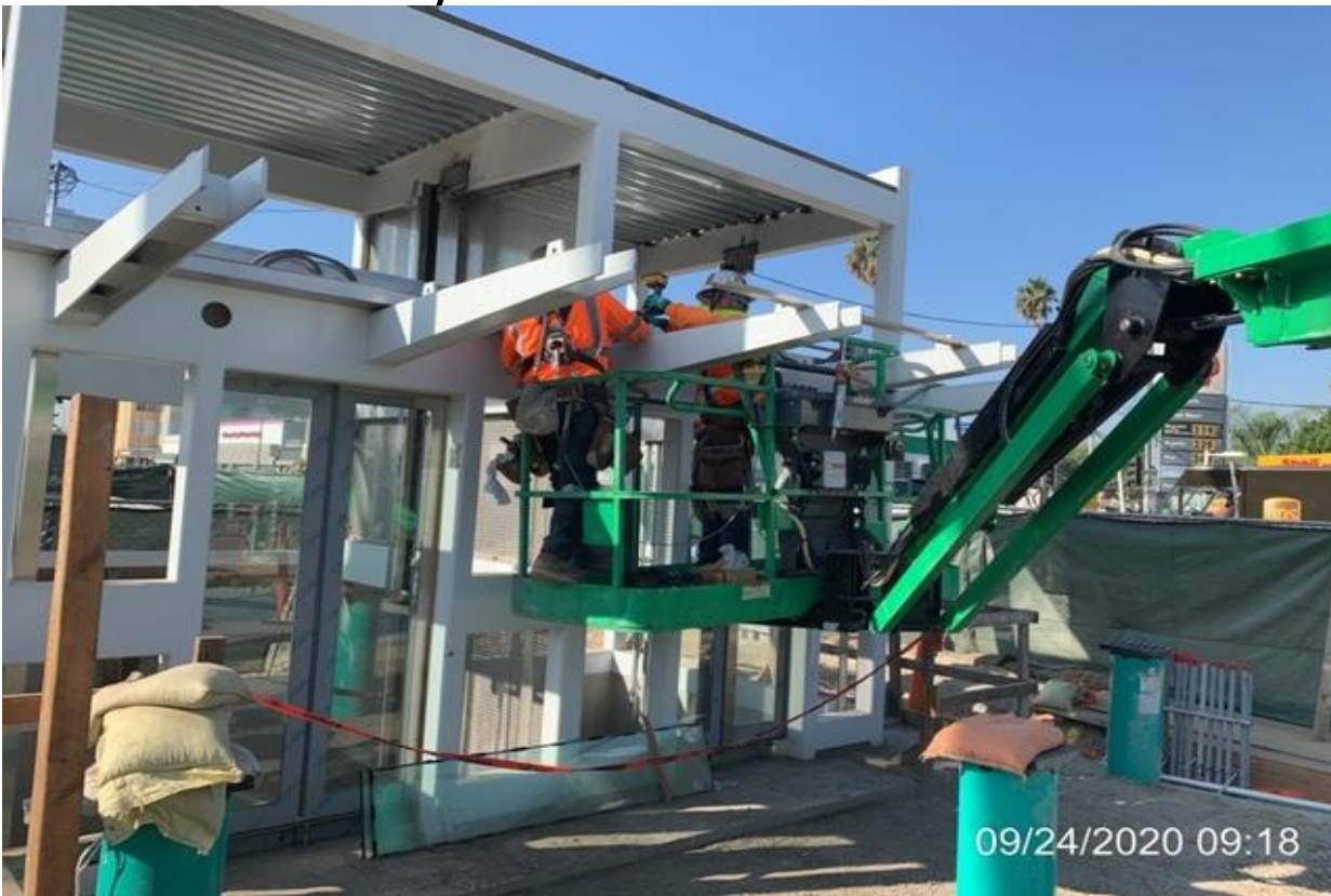
EXPO STATION SITE – Installing gutters and louvers to Elevators 1&2 at the plaza level.
