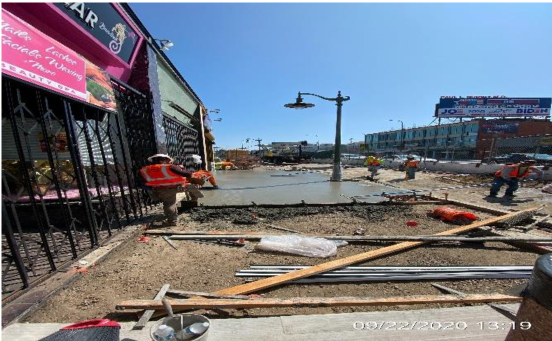
LEIMERT PARK STATION – Setting forms and concrete for new sidewalk panels on northbound Crenshaw Blvd near the far northwest corner of the plaza.
