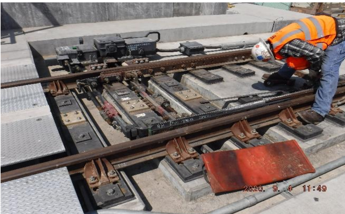
AVIATION/CENTURY- STA 70+11 TK#4/NB looking west – 10K1LHXO switch point manganese insert adjustment (Century)
