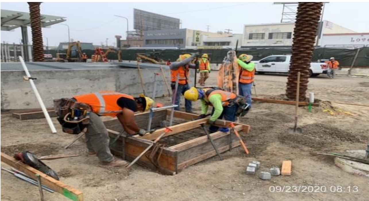
MLK STATION – Building formwork for the south map case and digging for the adjacent plumbing vent stack at the plaza level.
