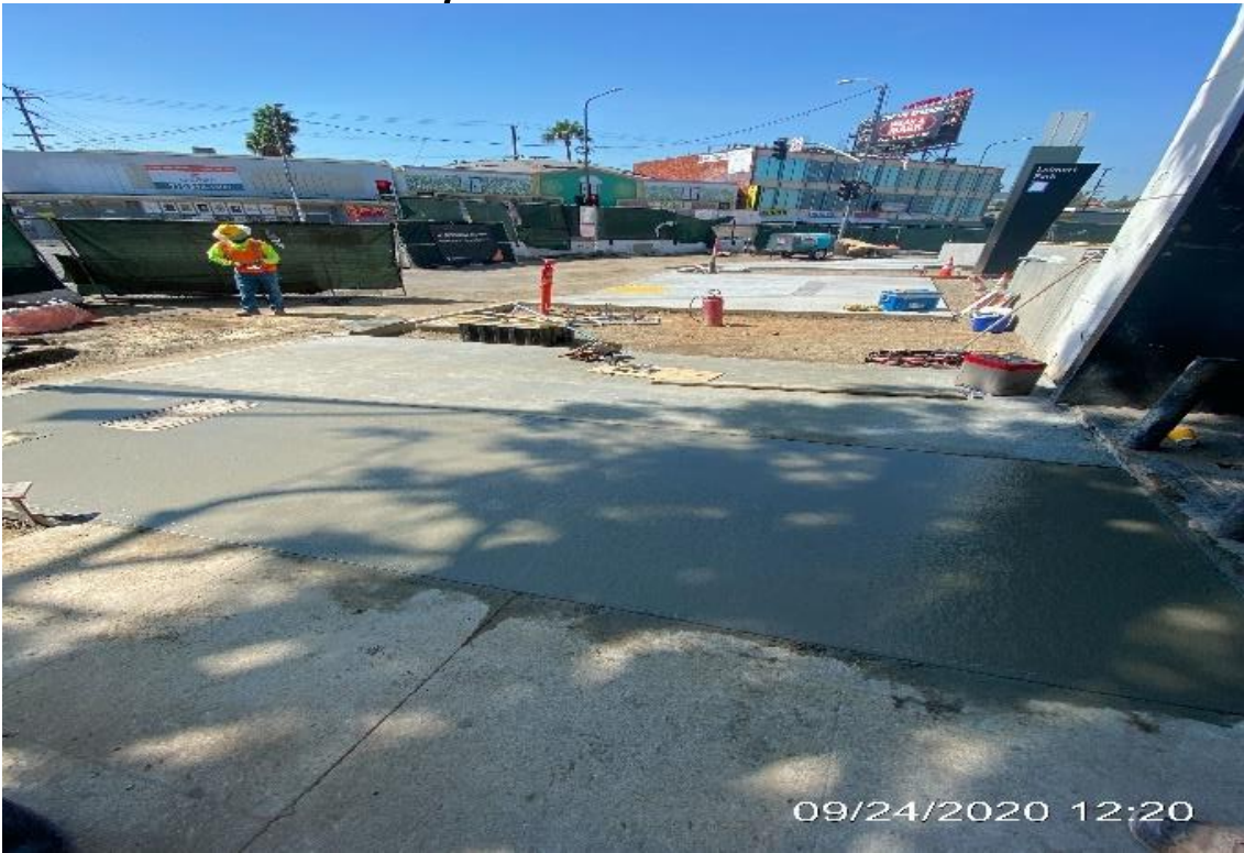
LEIMERT PARK STATION – Continue placing concrete for the new sidewalk along the far northeast corner of Crenshaw Blvd and 43rd Pl.
