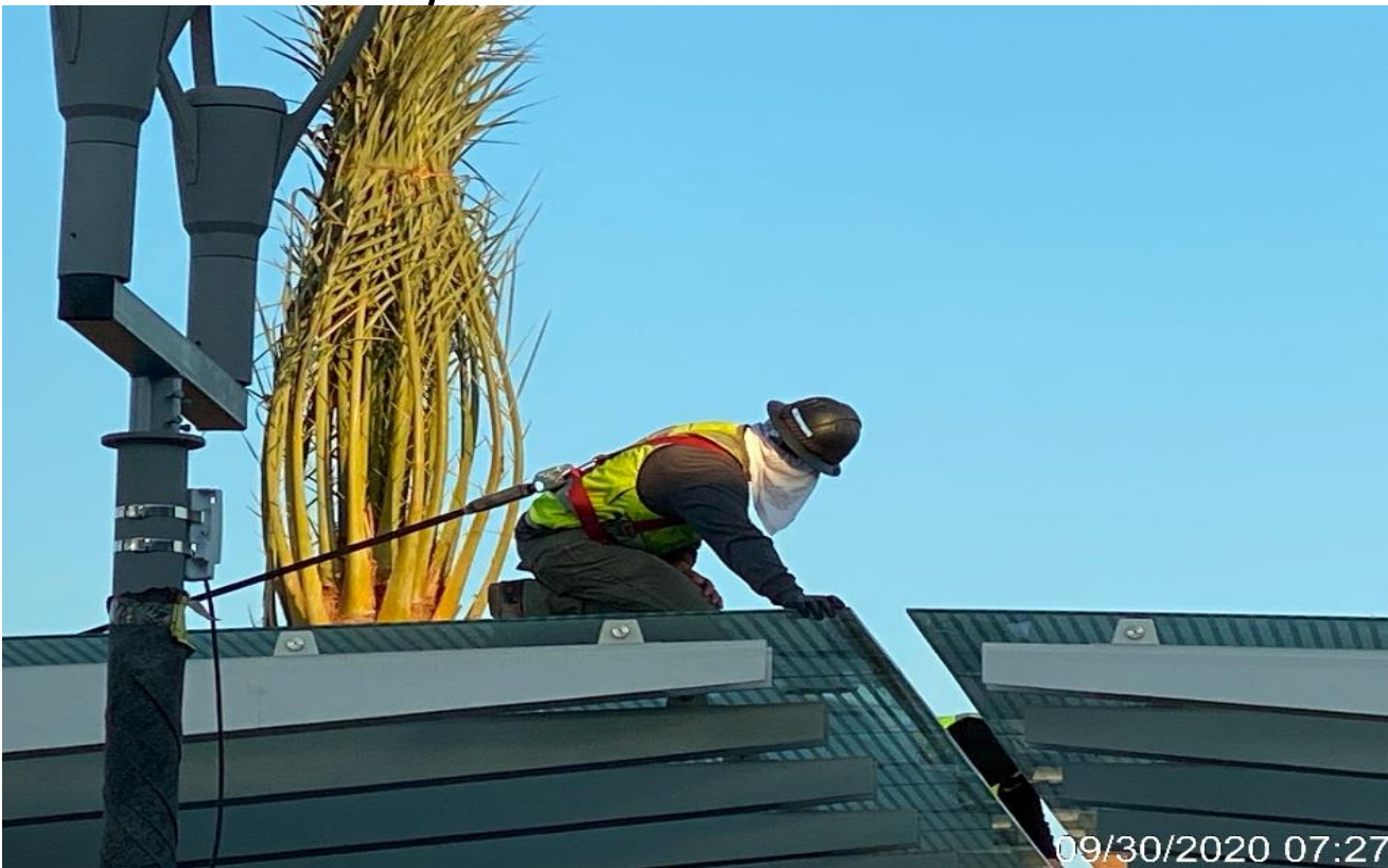
LEIMERT PARK STATION – Caulking and sealing expansion joints for the glass roof of the main entrance canopy at the plaza level.
