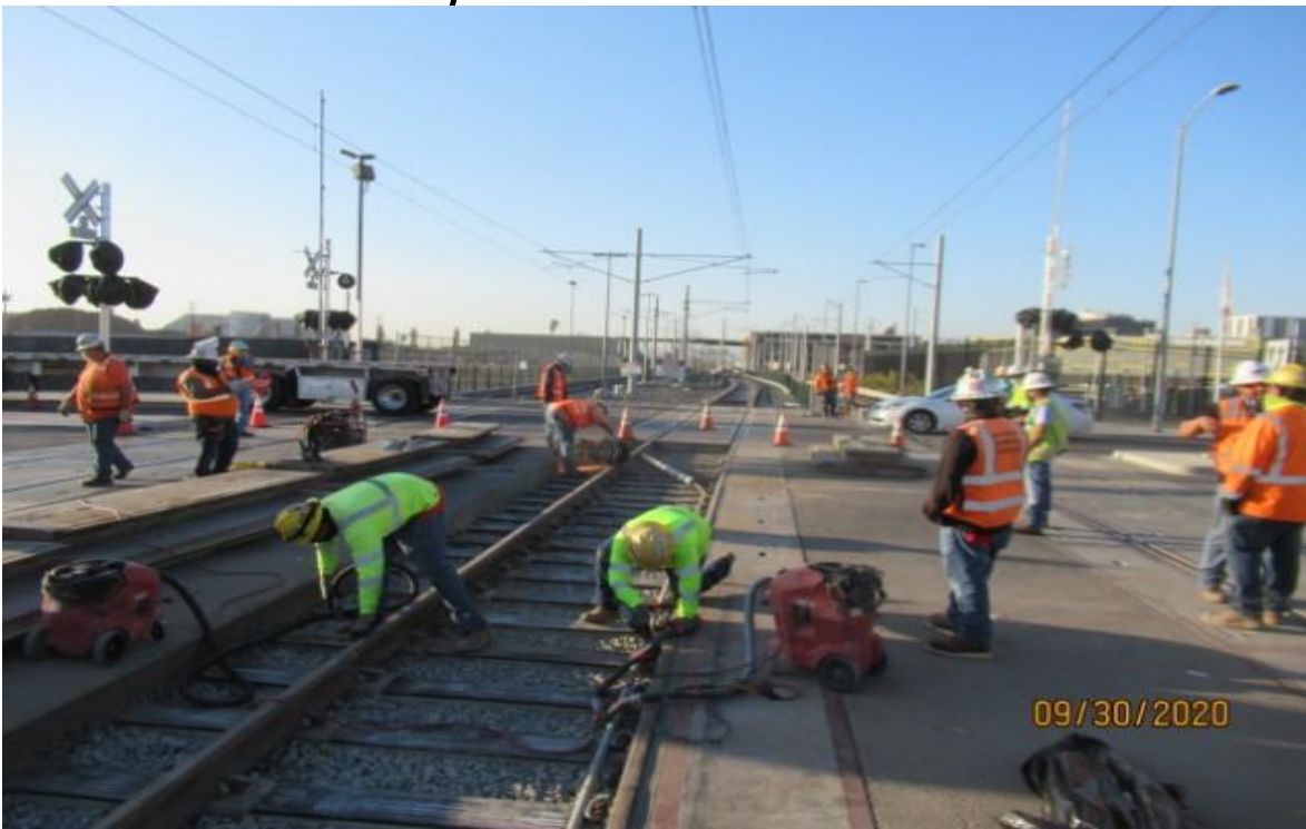
Arbor Vitae- LKC removing system loop O-bonds inside Arbor Vitae grade crossing SB track between STA 93+77 & 94+33 (looking south) Rework RFI-01499
