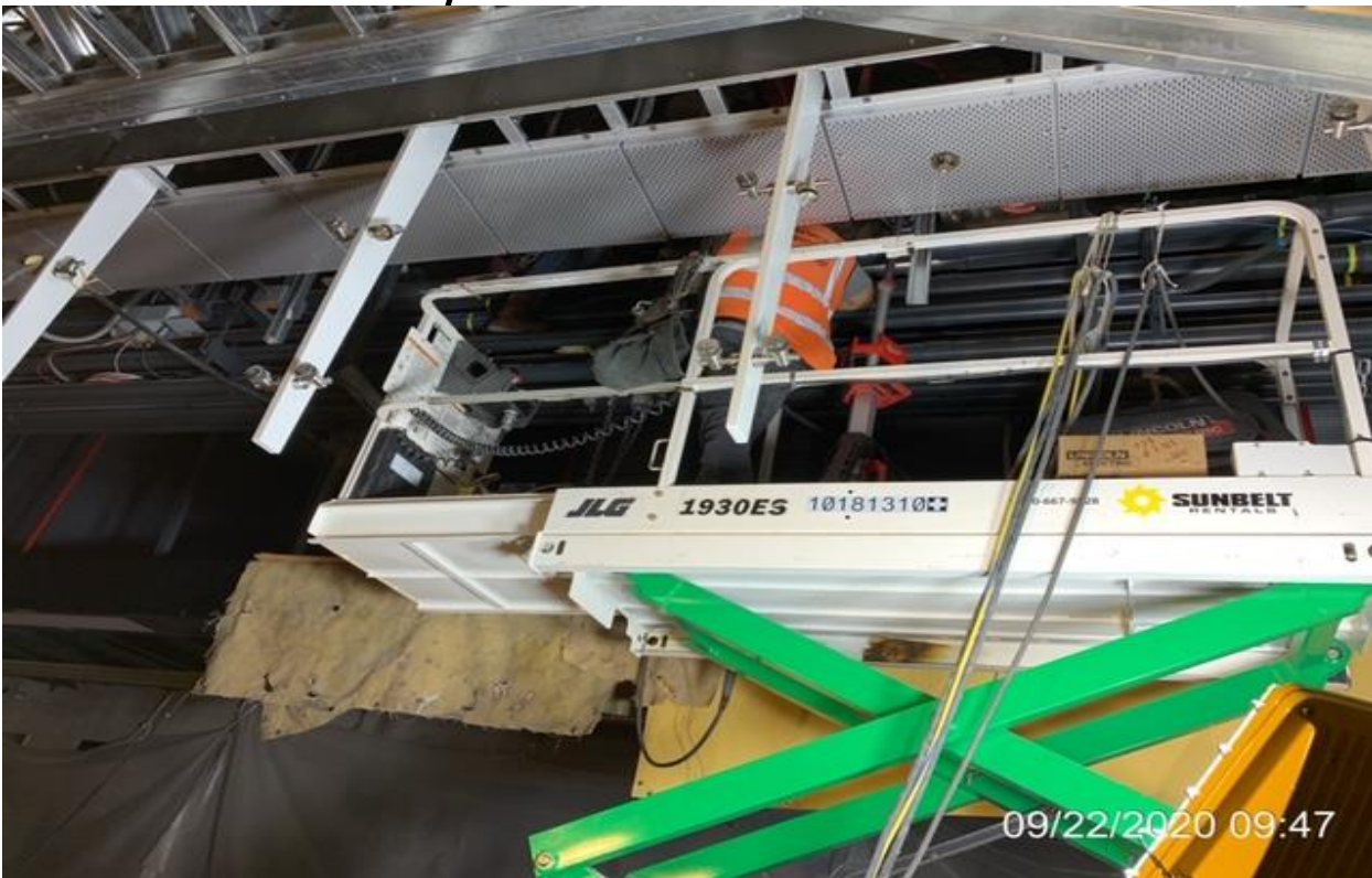
MLK STATION – Installing support arms for the LCD/LED variable messaging sign system along the northbound platform level.
