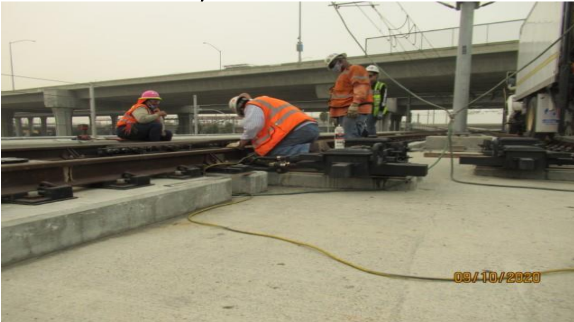
Guideway- HCC Foreman evaluating condition of right (straight) side Switch Point on 0FRHXO NBW track POS STA 15+98 GL Wye (looking southeast) Rework for damaged Switch Point repair
