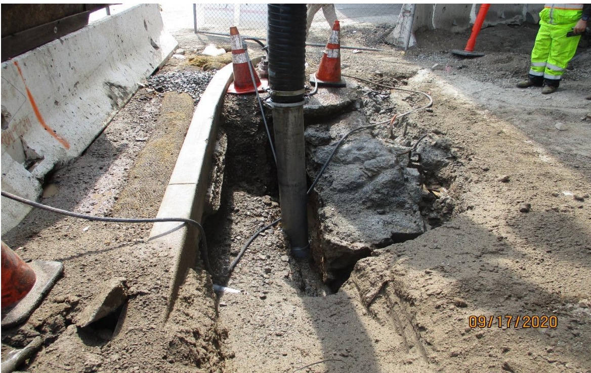
104 th street- Obstruction found during traffic signal conduit installation at the NW corner of Aviation and Century
