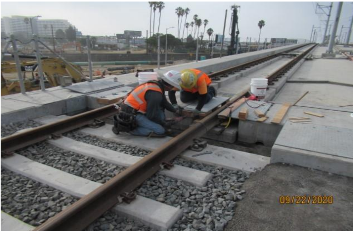
AVIATION/CENTURY- WSCC setting grout forms on Emergency Walkway Crossing foundations NB track Century/Aviation Bridge STA 74+65
