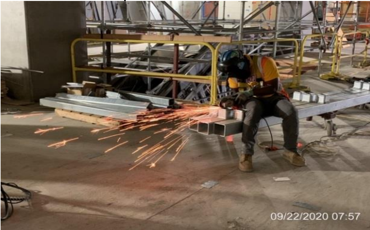
EXPO STATION – Fabricating grid support system and installing base plates for the mosaic art wall at the concourse level.
