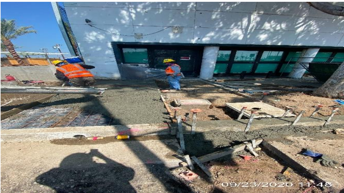
LEIMERT PARK STATION – Installing formwork and placing concrete for new sidewalk along the far northeast corner of Crenshaw Blvd and 43rd Pl.
