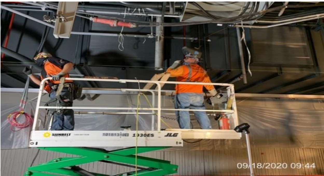
MLK STATION – Continue welding down stand support poles on the southbound platform level.
