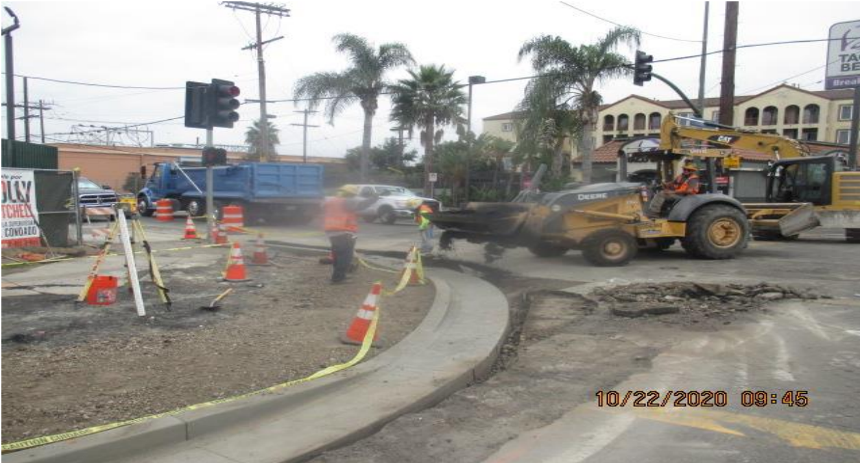
PARK MESA – Continue excavating to extend sidewalk on the northeast corner of Crenshaw Blvd and 60th St.
