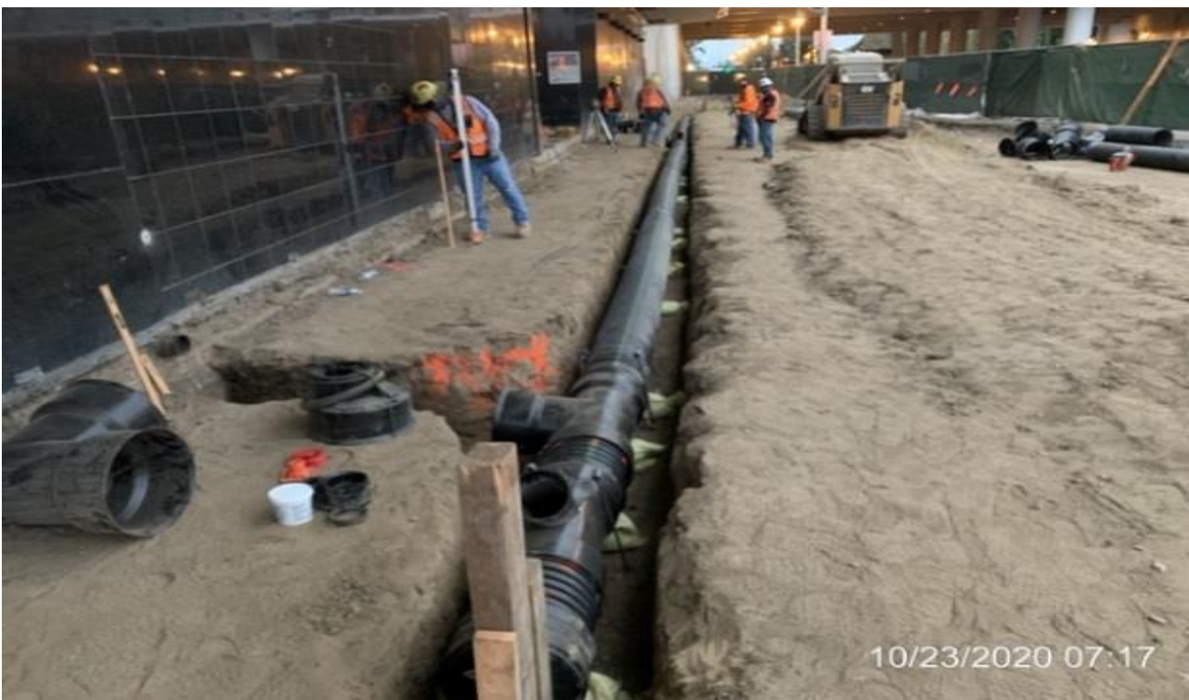
MLK STATION – Continue laying down HDPE pipe for the mall roof drainage at the far northwest area of the plaza.
