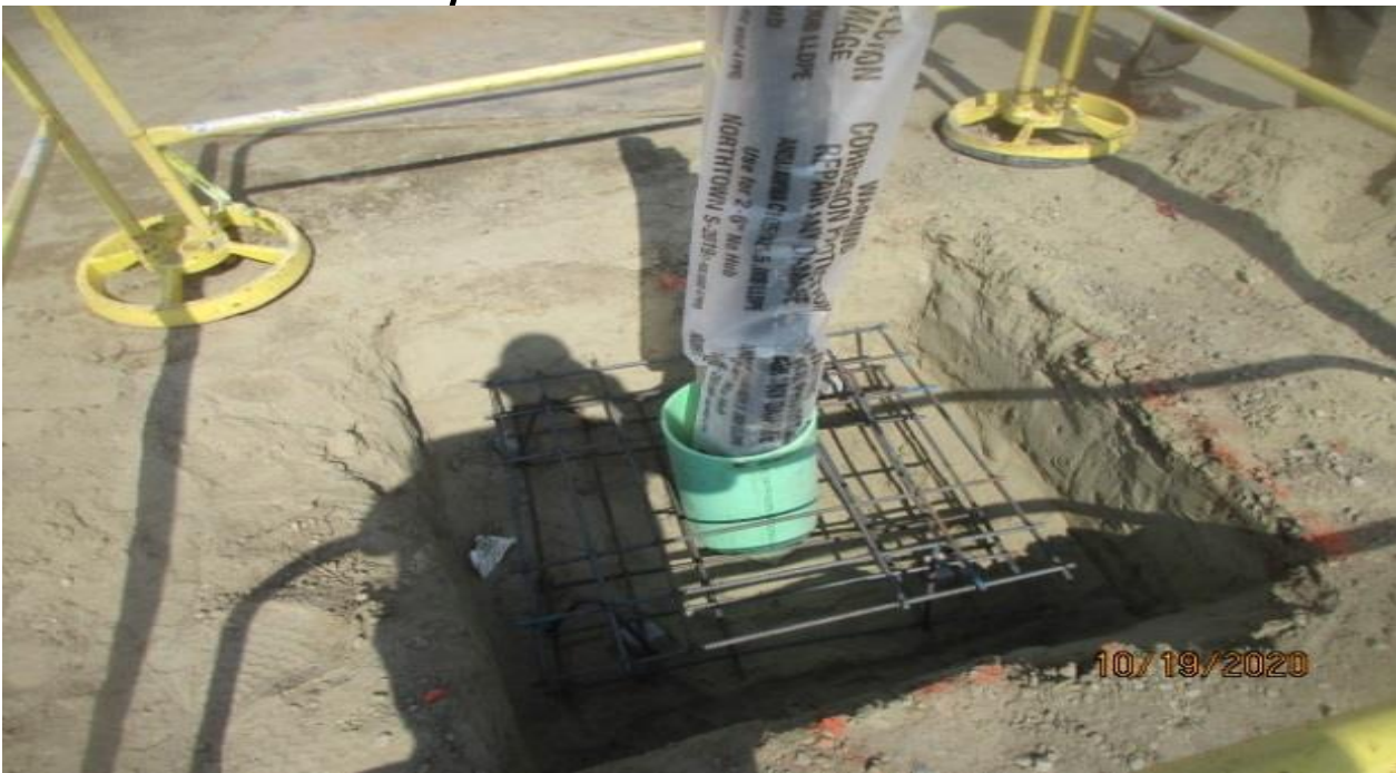
MLK STATION – Setting rebar for the south vent stack foundation at the plaza.
