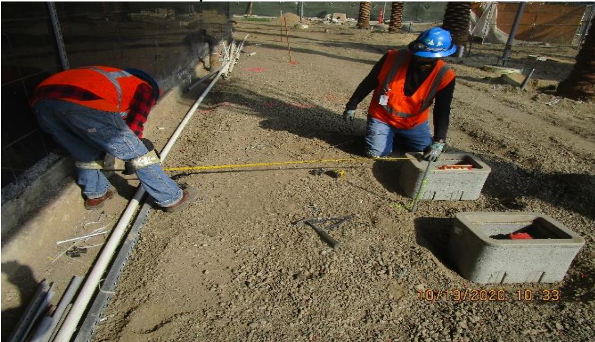
MLK STATION – MLK Plaza, North plaza continued setting embedded comm & lighting pull boxes to finish concrete elevation.
