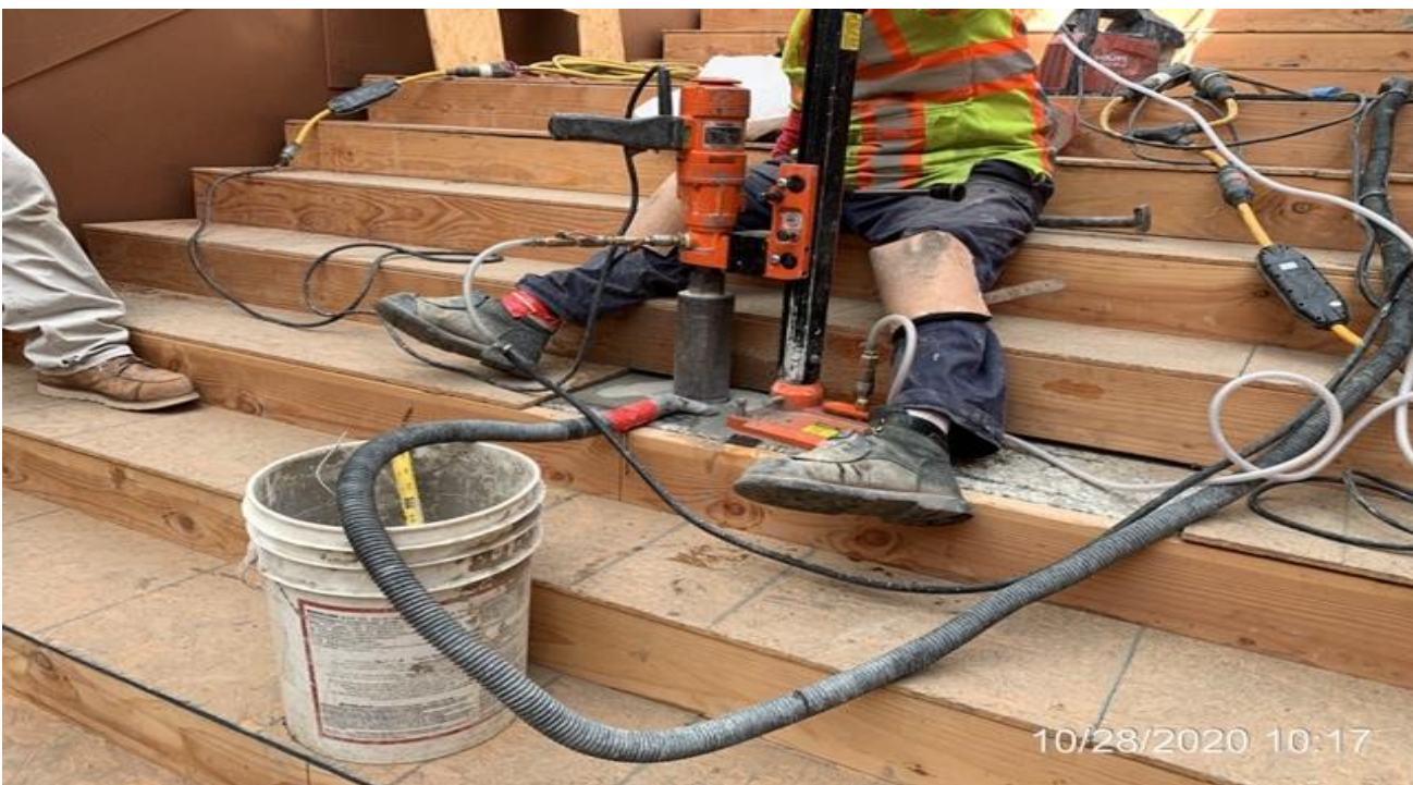
MLK STATION – Coring through Staircase #1 for handrail installation from plaza to concourse.
