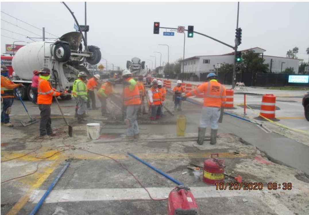
PARK MESA – Continue placing slurry on the north and southbound lanes for restoration at the intersection of Crenshaw Blvd and 57th St.
