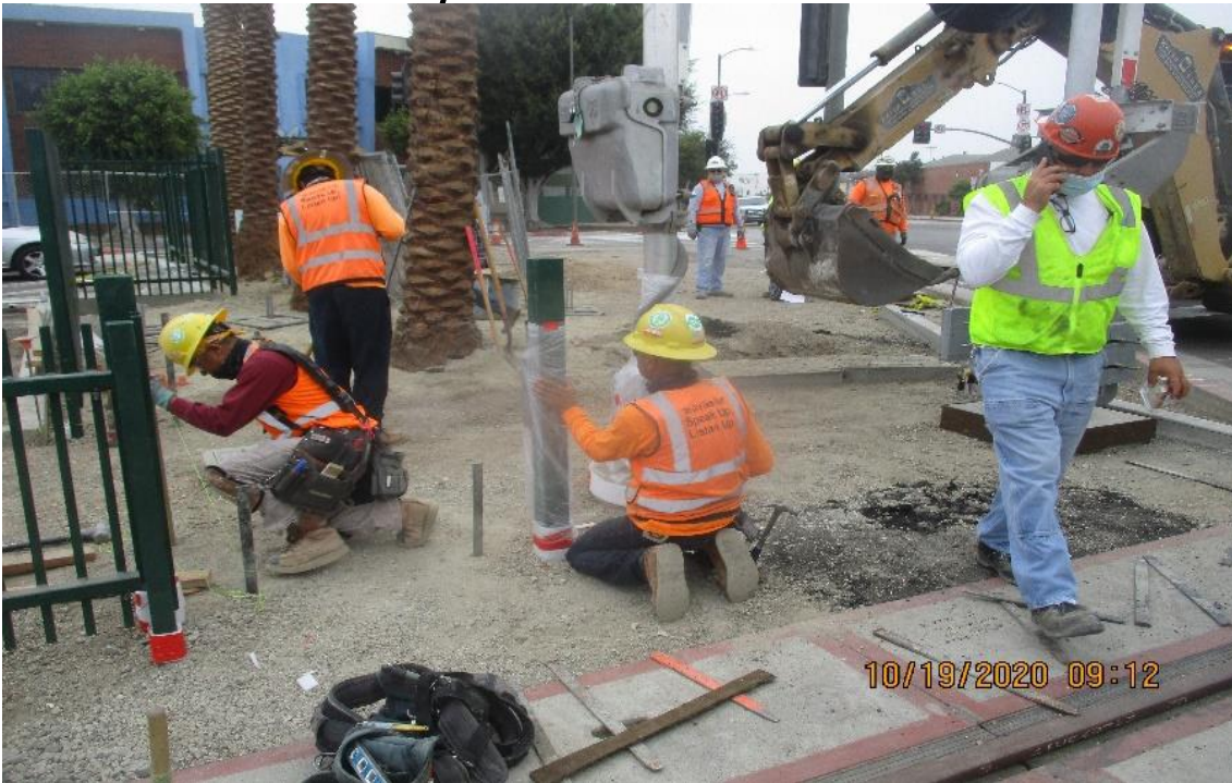
AVIATION/CENTURY- WSCC Excavated, made grade for and placed SWK conc at West St crossing.
