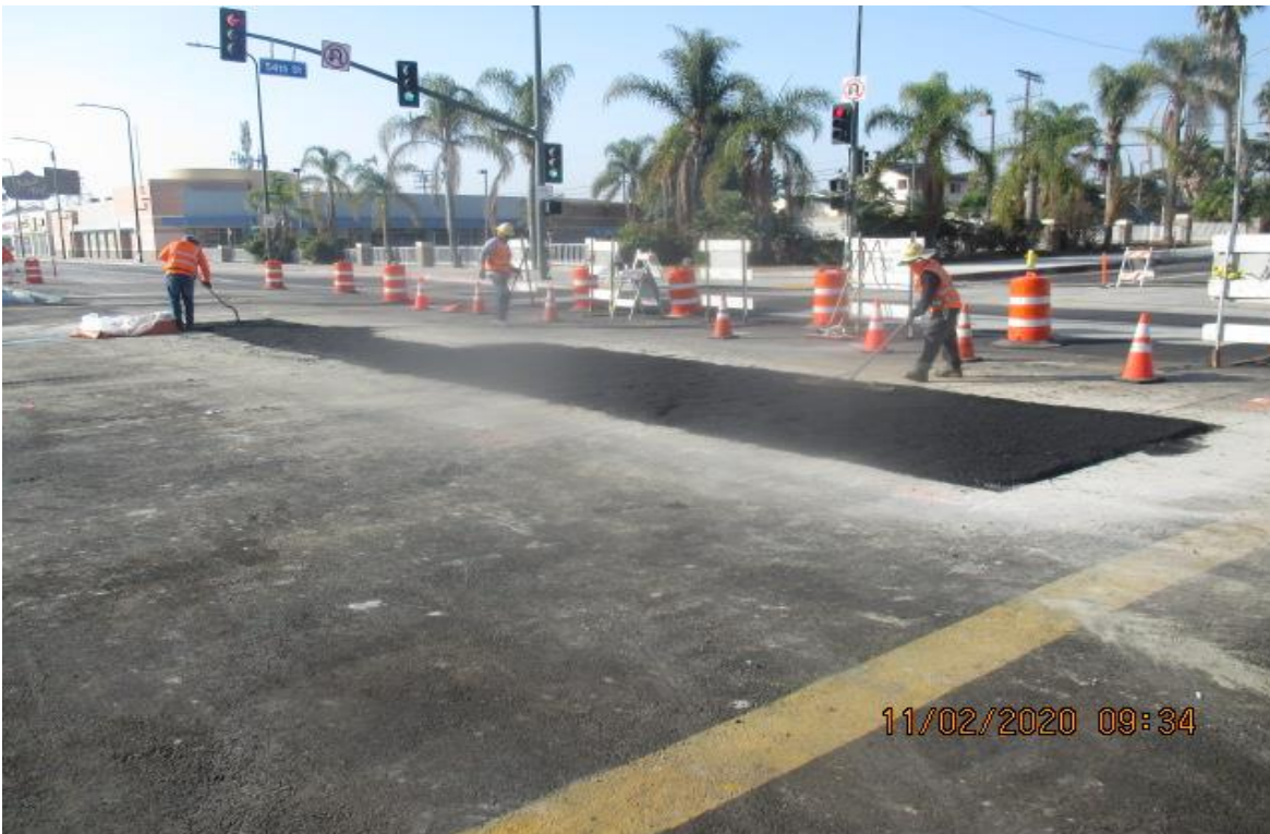
PARK MESA – Placing asphalt concrete for road slab on the intersection of Crenshaw Blvd and 54th St.
