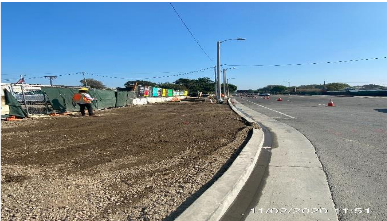
EXPO STATION SITE– Continue excavating/grading sidewalk on westbound Obama Blvd and Crenshaw Blvd.
