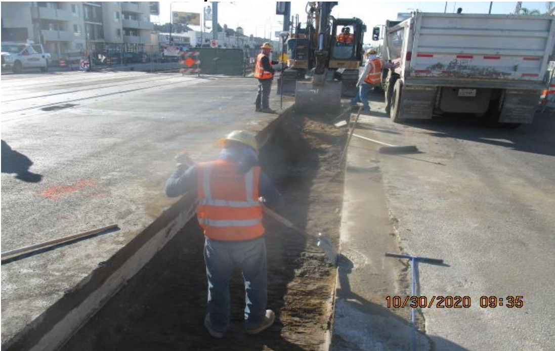
PARK MESA – Excavated and removed existing road slab on the intersection of Crenshaw Blvd and 54th St.
