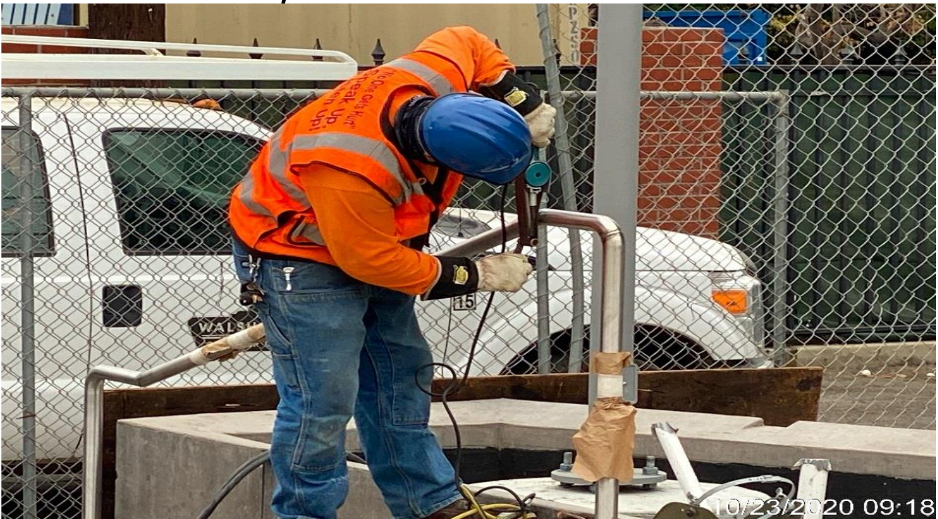
LEIMERT PARK STATION – Modifying handrails for the east entrance stairs at the plaza.
