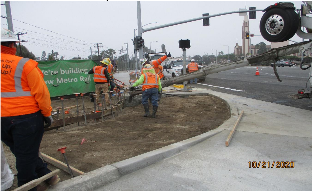
La Brea – Placing concrete for the ADA ramps at the La Brea Station.
