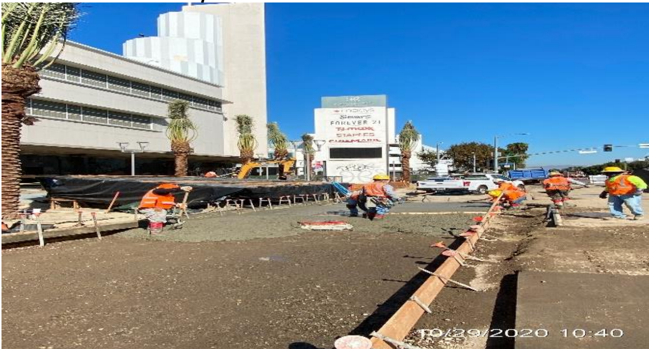
MLK STATION – Placing concrete along the east side of the plaza for new curb/gutter and bus pad installation.
