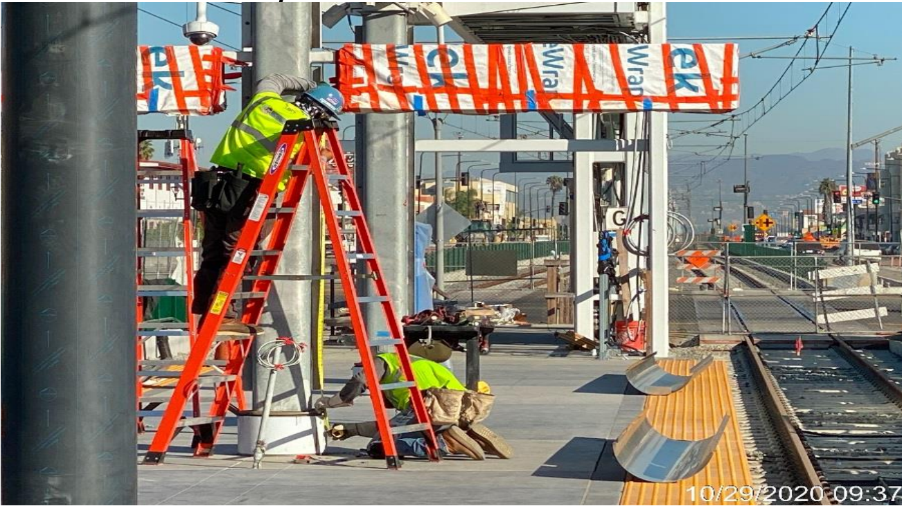
HYDE PARK STATION – Continue installing stainless steel cladding covers for the platform columns.
