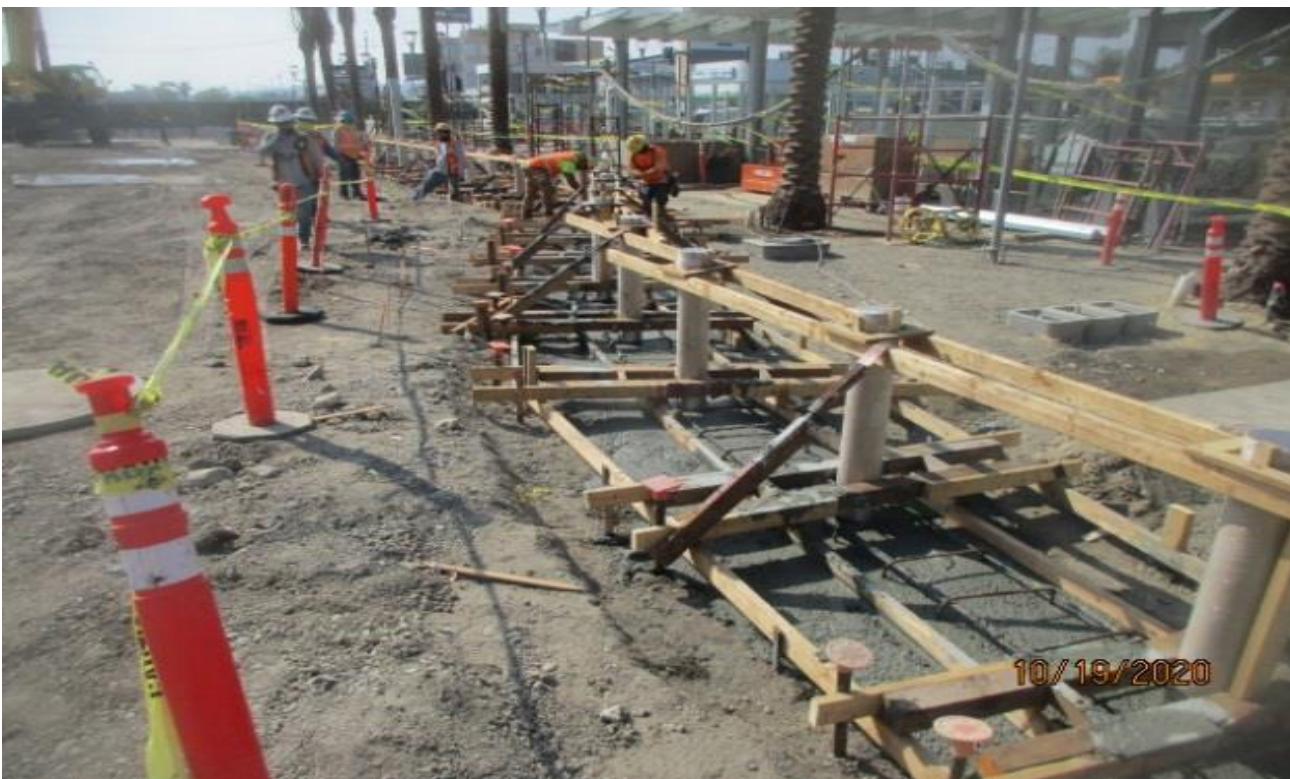
EXPO STATION – Continue building formwork and setting the east side bollard foundations at the plaza.
