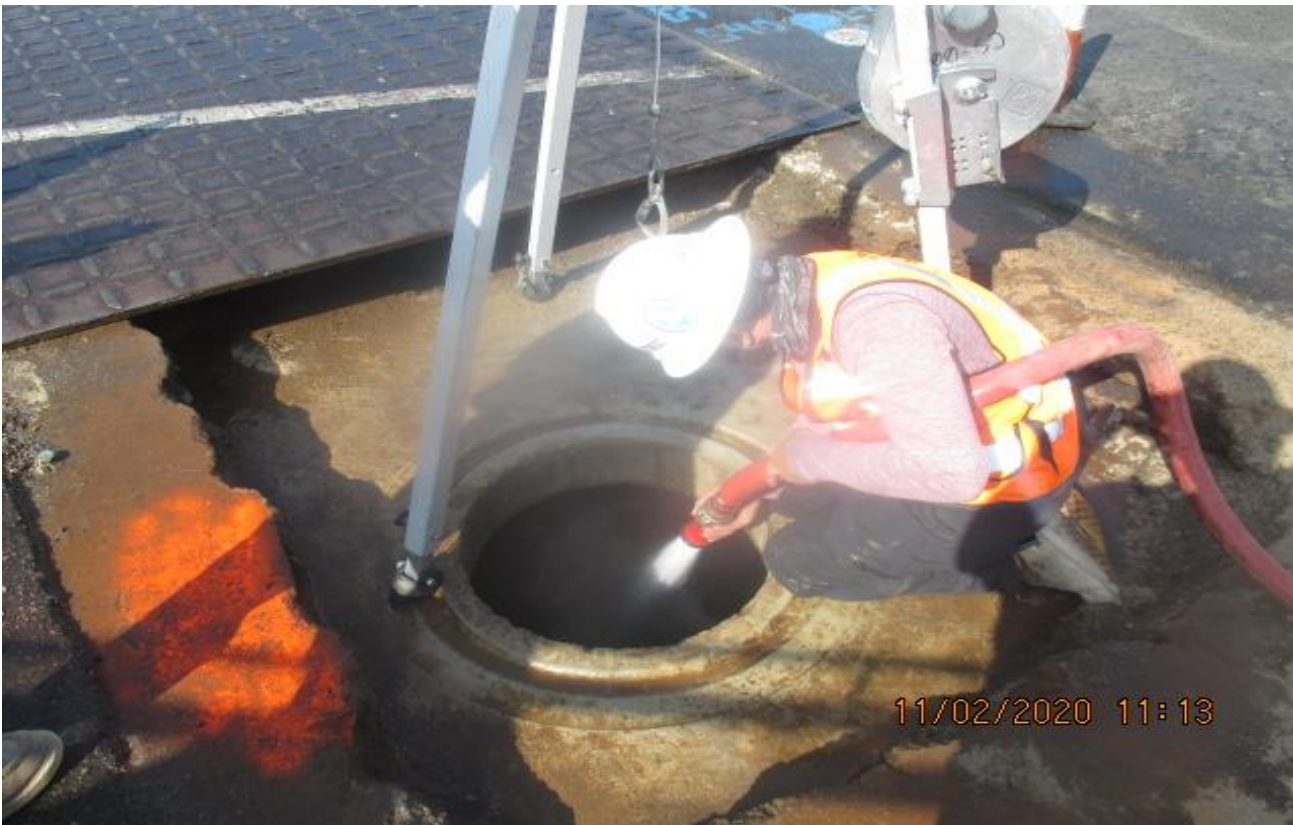
PARK MESA – Sacking and patching Manhole #20 on northbound Crenshaw Blvd and 60th St.
