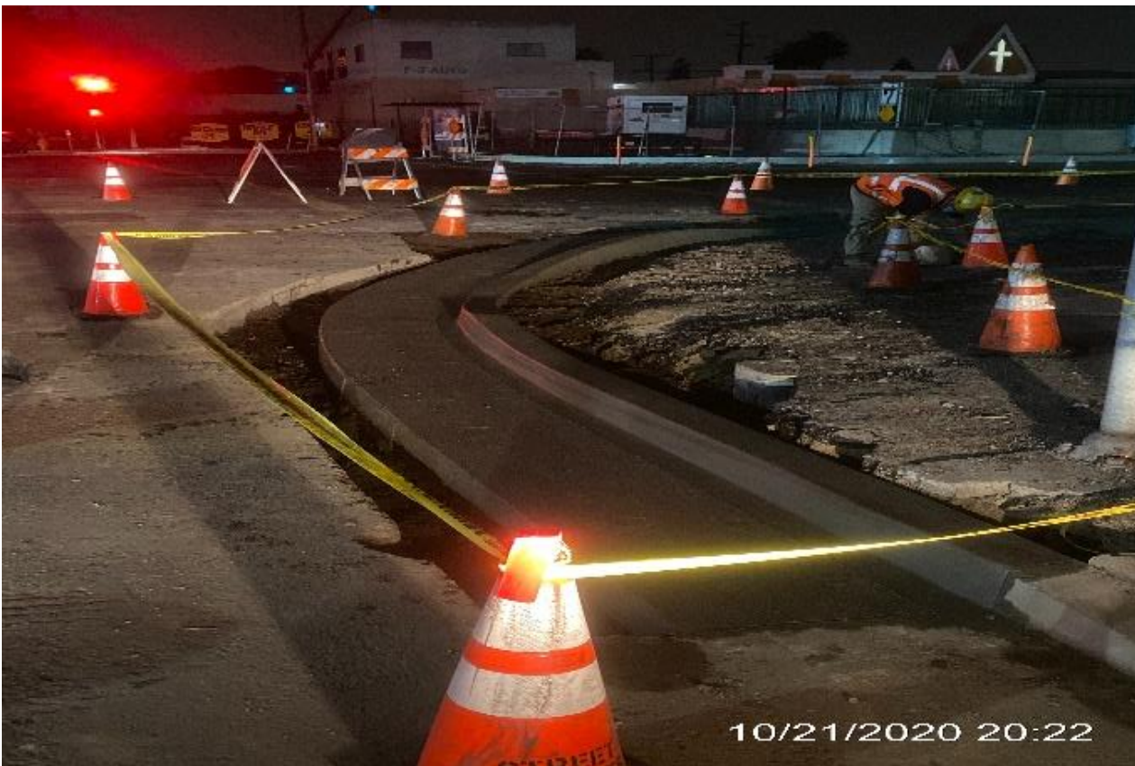
PARK MESA – Built formwork and placed concrete for the new curb and gutter installation on the northeast corner of Crenshaw Blvd and 60th St.
