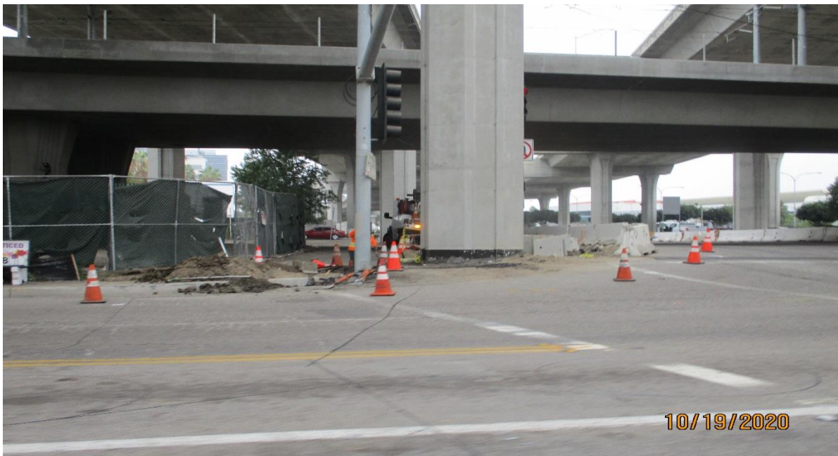
AVIATION/CENTURY- Trenching for the traffic signal conduit on the SW corner of Aviation and Imperial.
