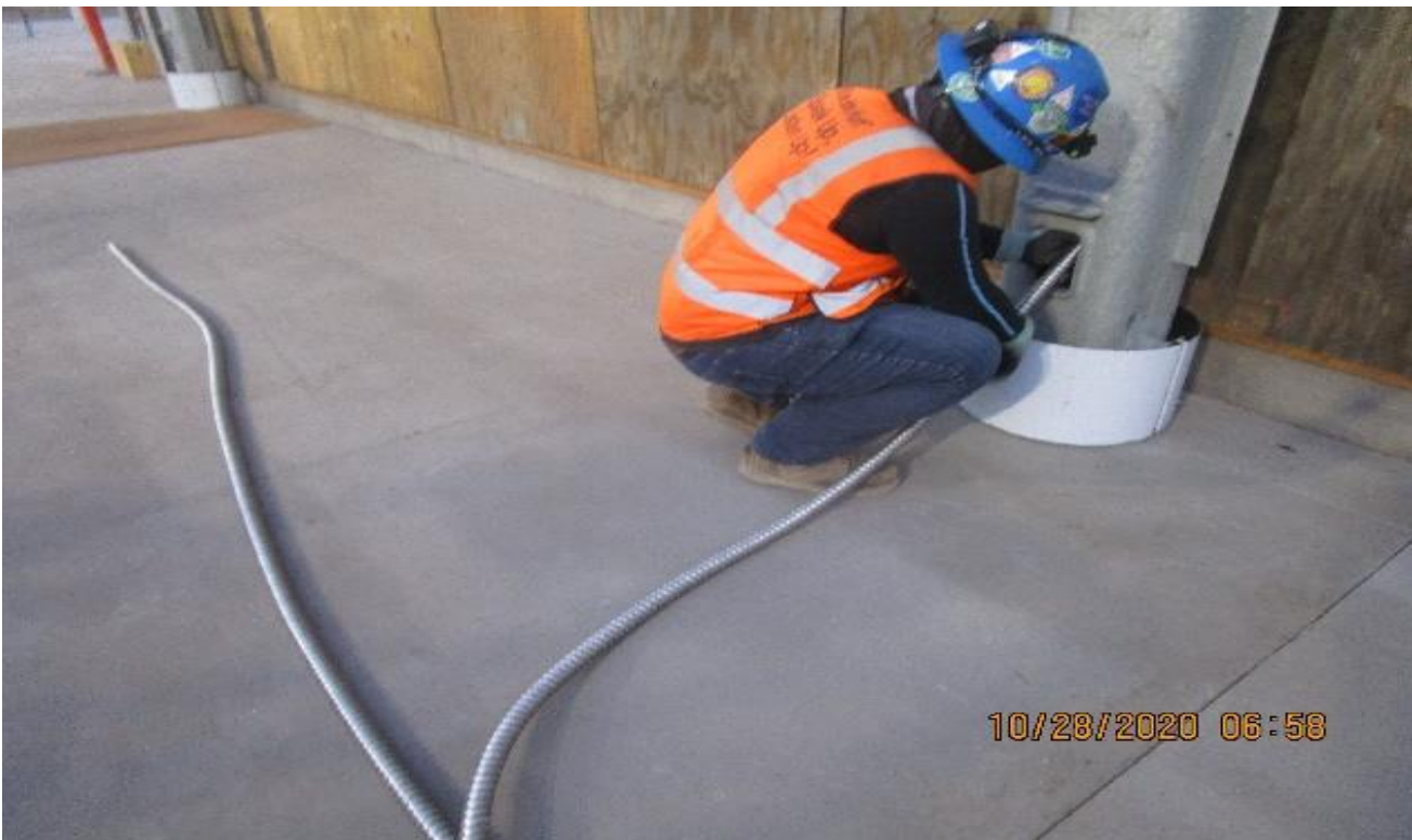
LEIMERT PARK STATION – Roughing flex to the main entrance canopy columns for BOCA light fixtures at the plaza.
