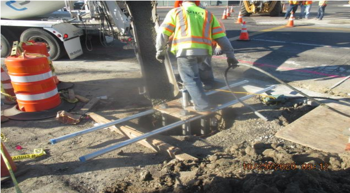
PARK MESA – Excavating for the installation of power conduits for signal lights and placing concrete on northbound Crenshaw Blvd and 60th St.
