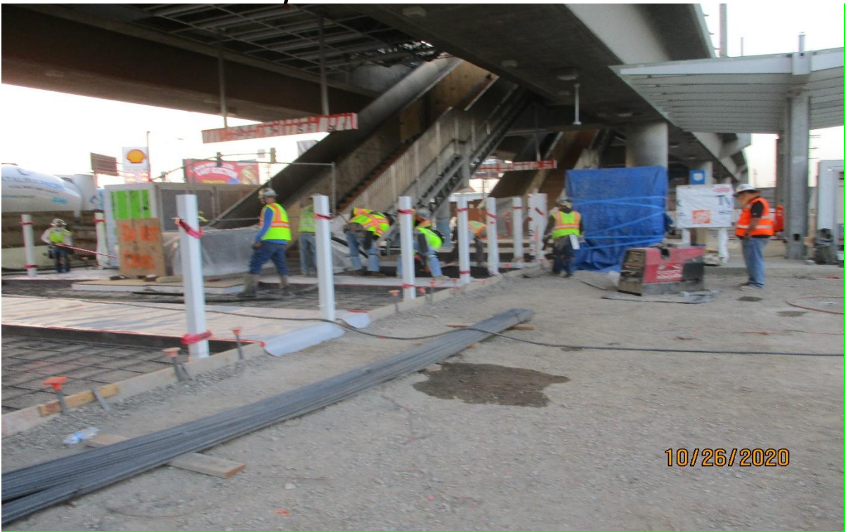
AVIATION/CENTURY- Placing concrete for the stairway and escalator landing area at the Aviation Station.
