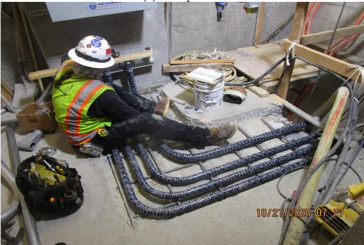
Crenshaw/Vernon – Vernon Platform, Sump pump room (N) T110 continued rough in controller GRC to pit (3) 1-1/2” & (2) 2”
