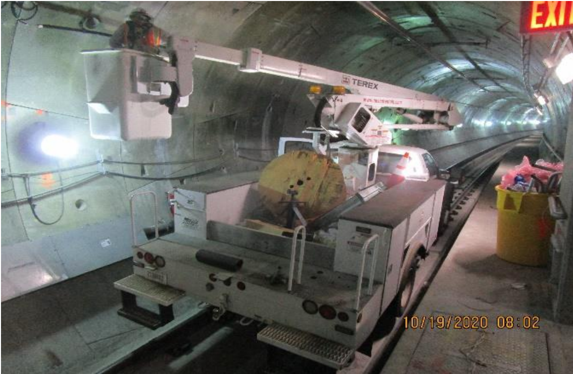
Crenshaw/Vernon – Southbound bored tunnel Vernon to MLK Begin removing 1-1.4” Radiax cable between CP5 & (S) MLK portal
