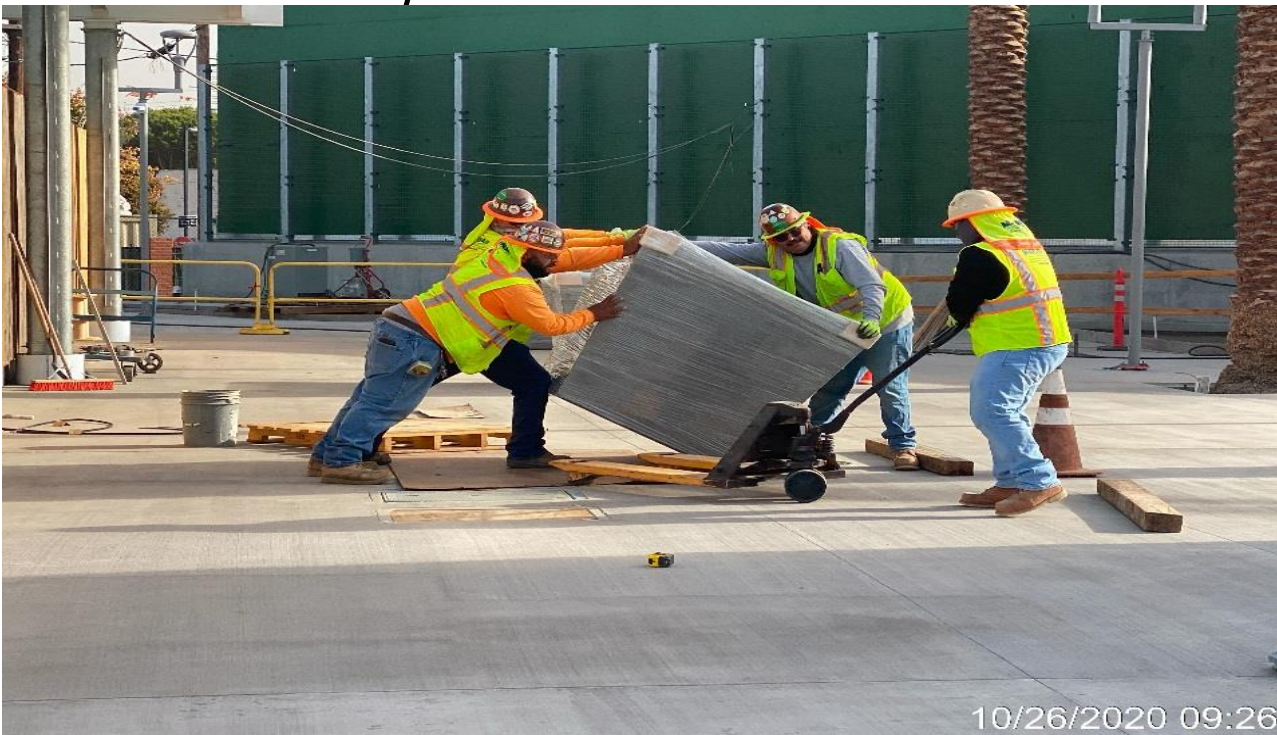
LEIMERT PARK STATION – Continue setting and installing planter pots throughout the plaza.
