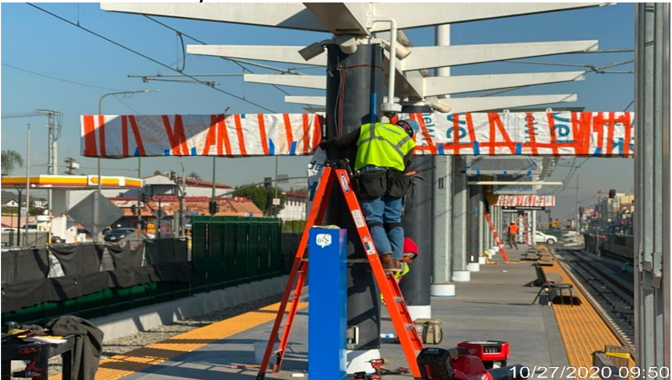
HYDE PARK STATION – Installing stainless steel cladding covers for the platform columns.
