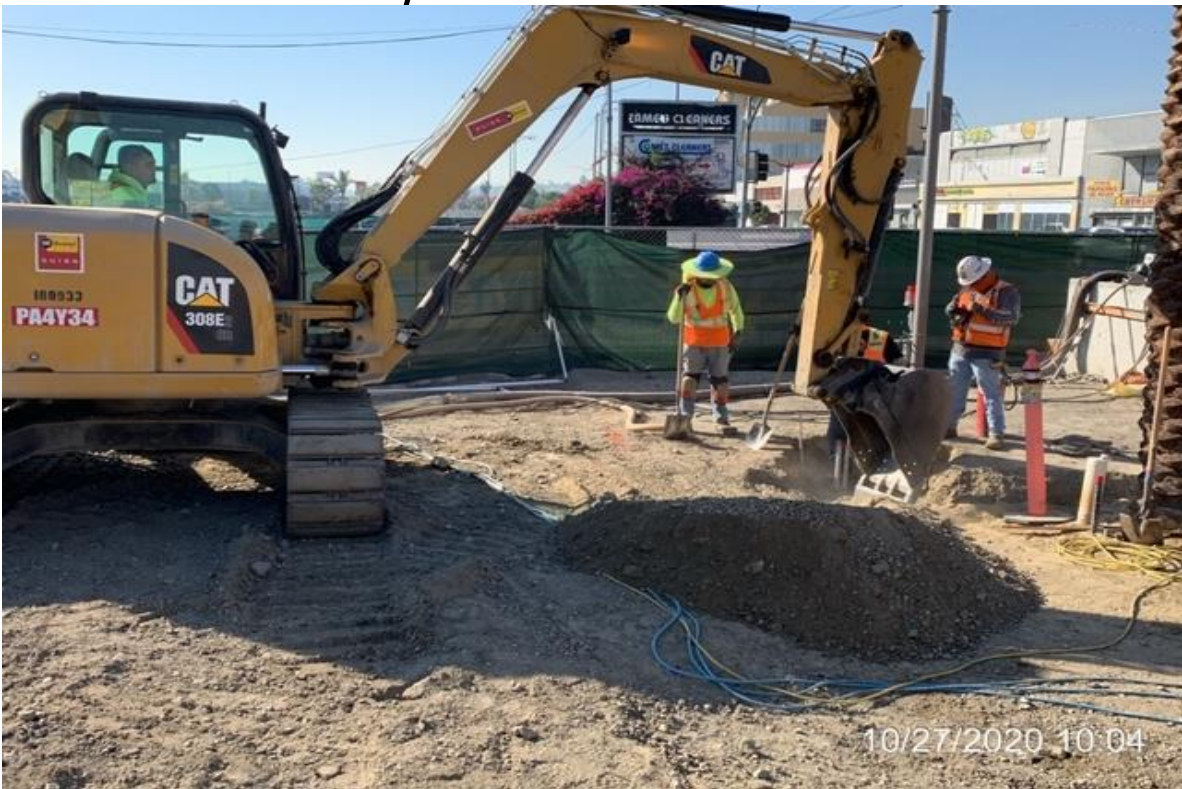
EXPO STATION – WSCC crew excavating to expose conduit for AT&T tie in.
