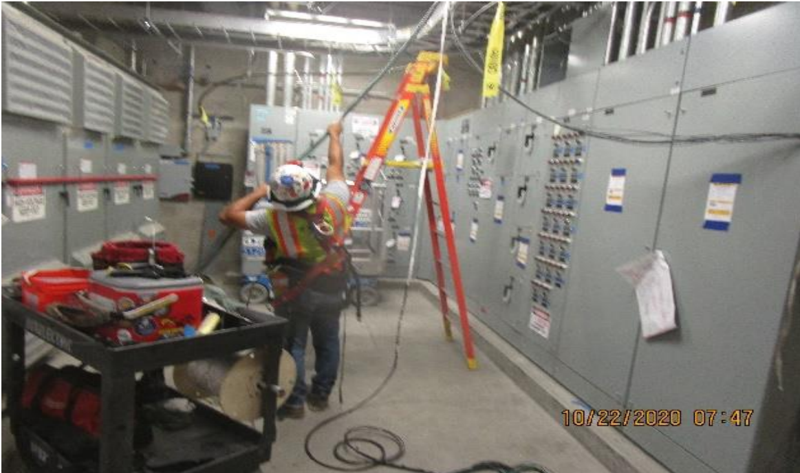
Crenshaw/Vernon – Vernon Concourse, Aux power (N) C119, MCC1/N (CIC) pulling #14 control wiring to PAC-6-2 mechanical damper
