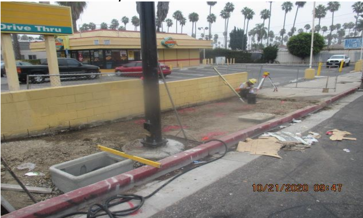
PARK MESA – Grading sidewalk in preparation for concrete placement on the northeast corner of Crenshaw Blvd and 48th St.
