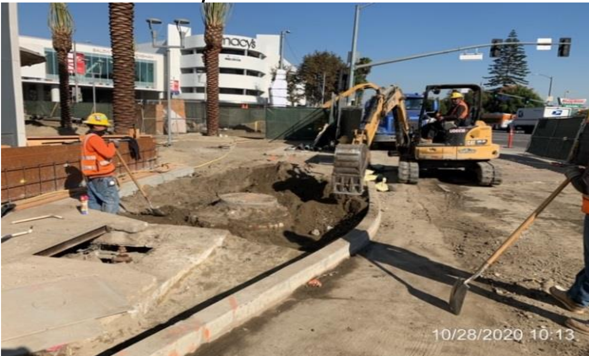
MLK STATION – WSCC crew grading north end of station adjacent to mall sign and planter.
