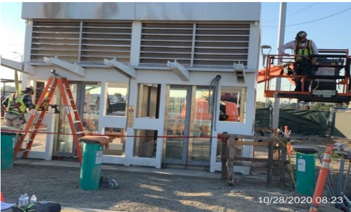
EXPO STATION – Giroux Glass fabricating and installing glass stops on elevator structure #1 and #2.
