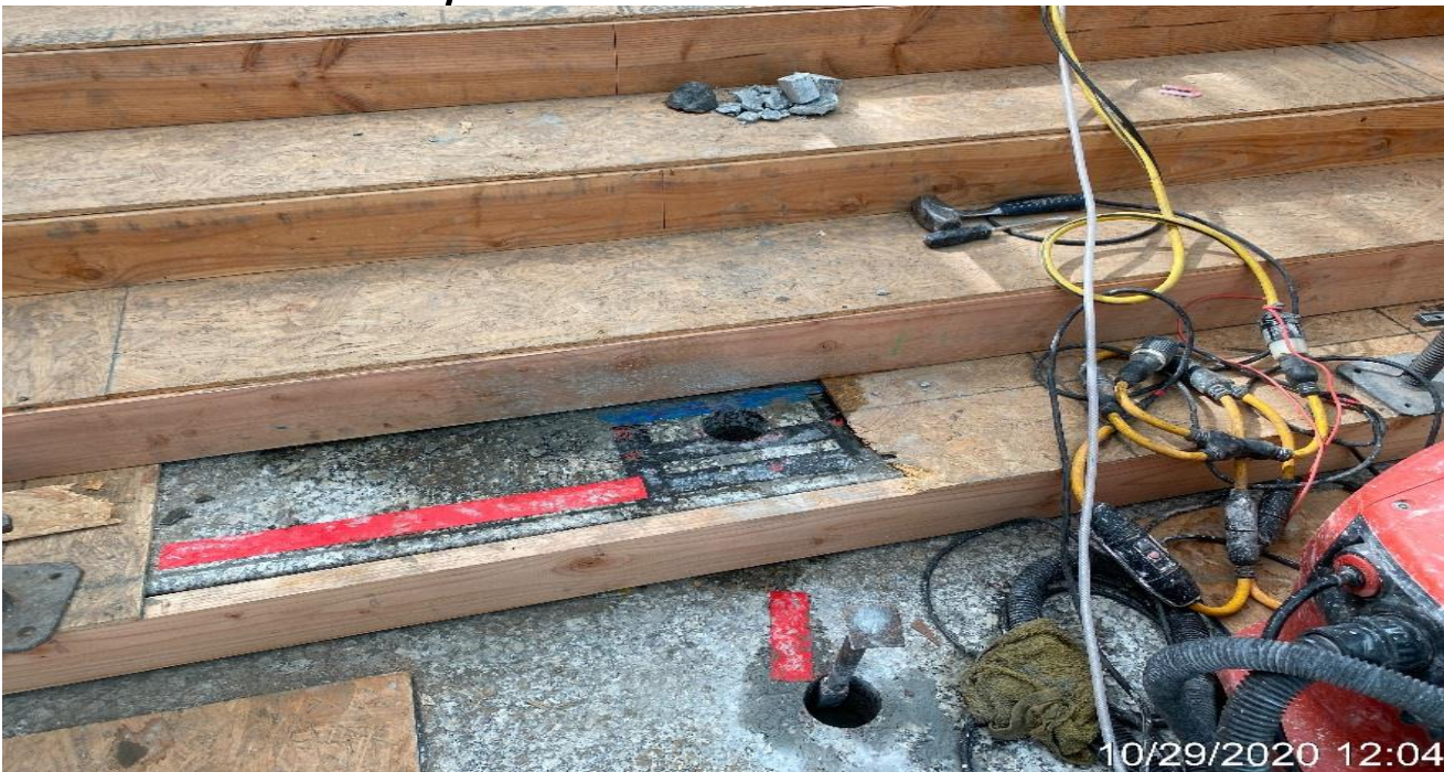
LEIMERT PARK STATION – Coring through Staircase #1 for handrail installation from plaza to the intermediate landing.
