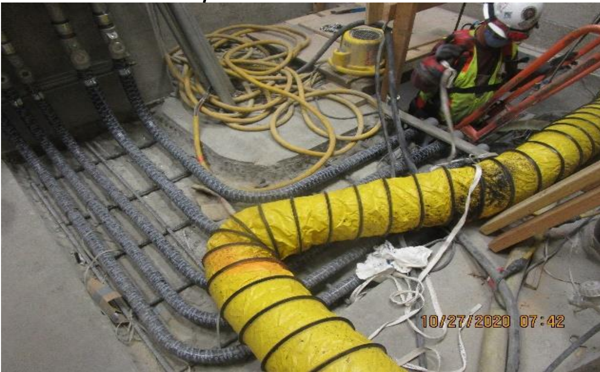
Crenshaw/Vernon – Vernon Platform, Sump pump room (N) T110 continued piping (3) 1-1/2" & (2) 2" GRC from control panel to pit
