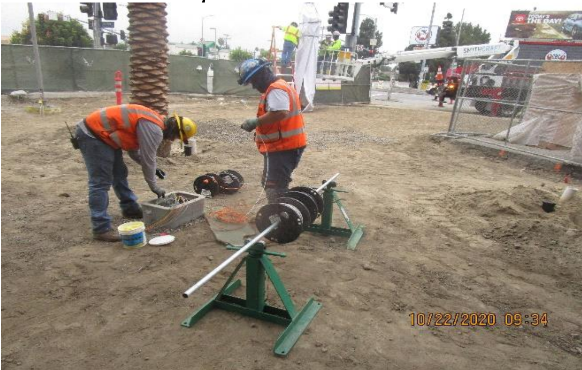
MLK STATION – MLK Plaza, North plaza continued pulling #10 XHHW-2's from embedded pull boxes to pedestrian light
