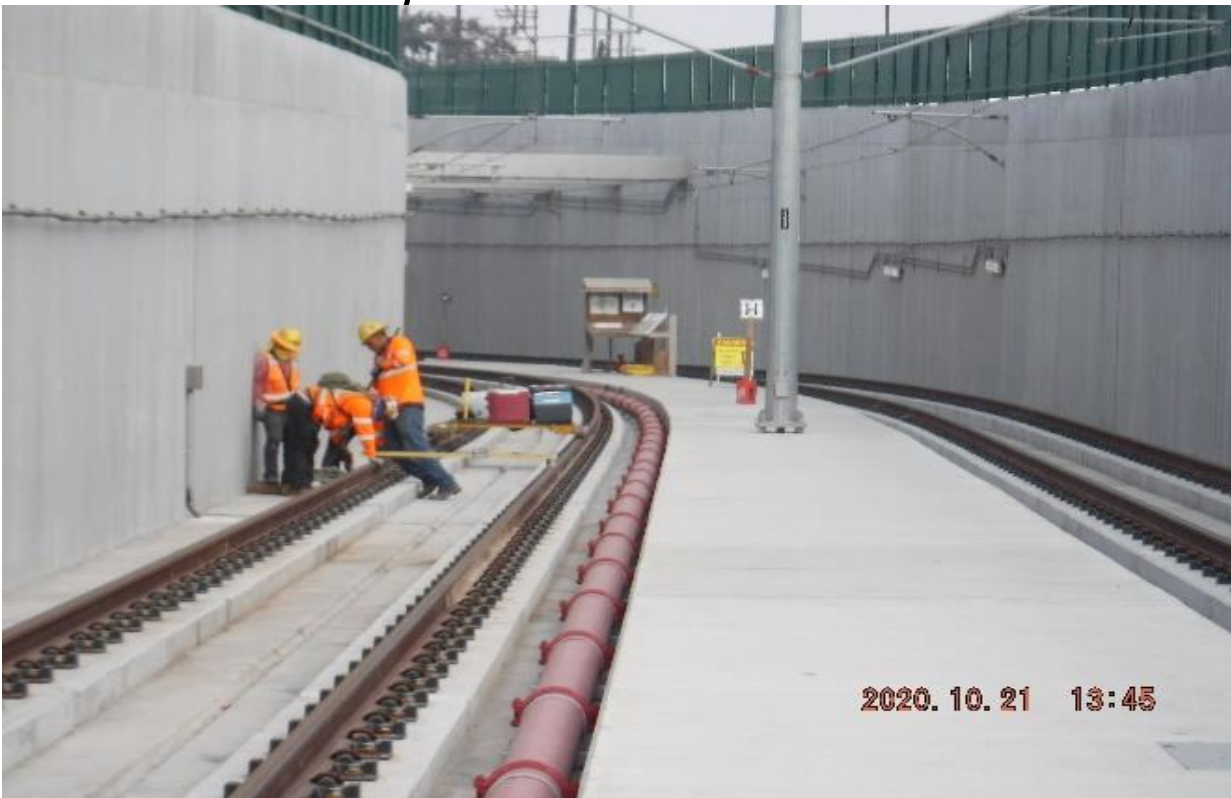
UG3 – STA 279+20 TK#3/SB looking north – UG3 (Victoria) checking track geometry and adjusting as needed (REWORK)
