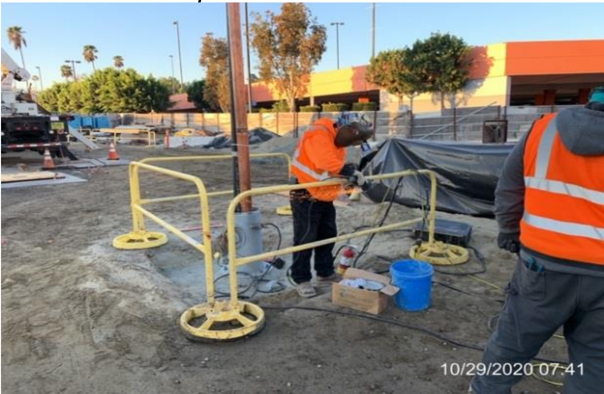
MLK STATION – Installing rebar to the north end planter wall footing at the plaza level.
