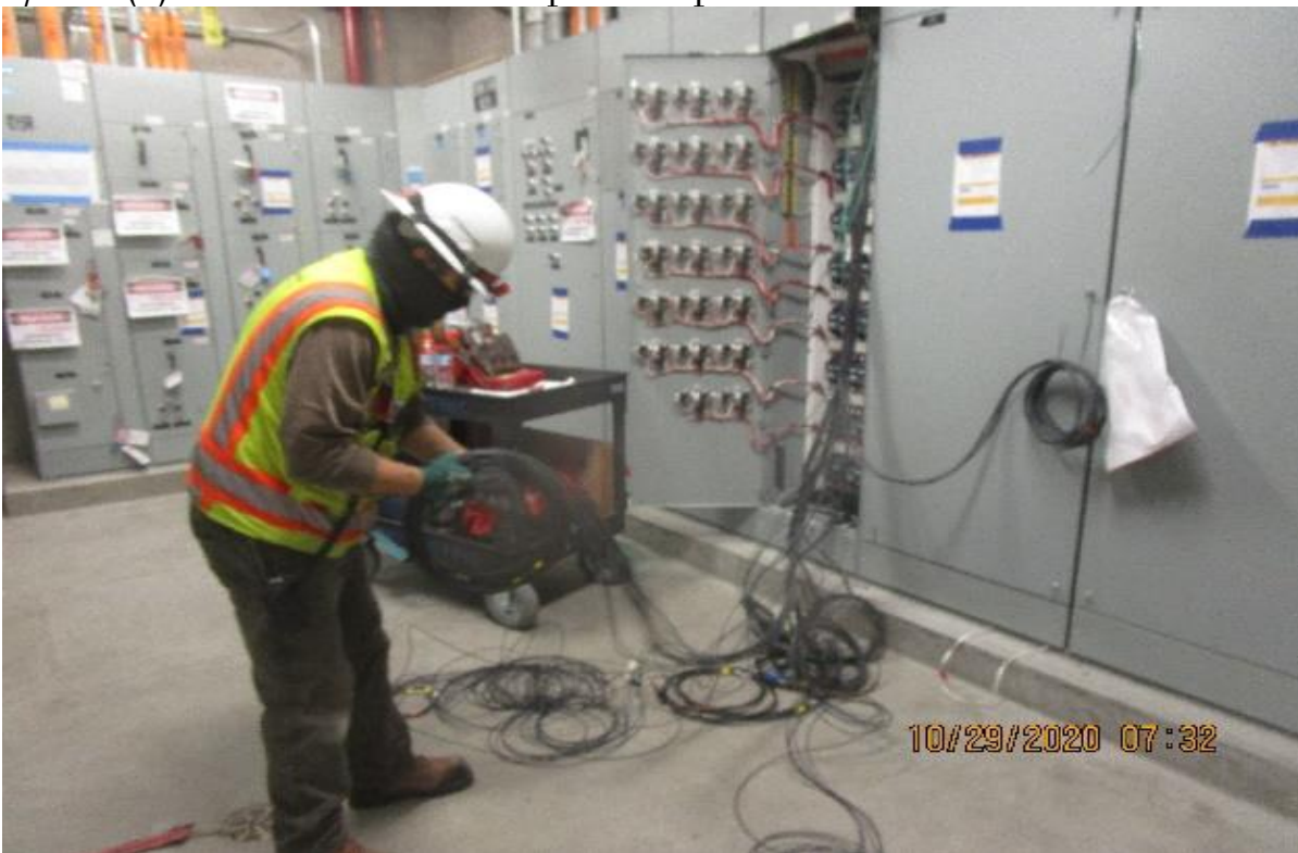
Crenshaw/Vernon – Vernon, Aux power (N) C119 continued identify, label & dressing FSD limit switch control #14 wiring MCC2/N
