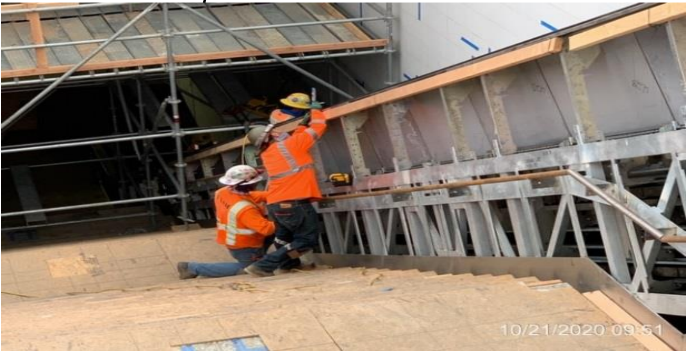
EXPO STATION – Continue excavating/trenching for the west side bollard foundations at the plaza level.
