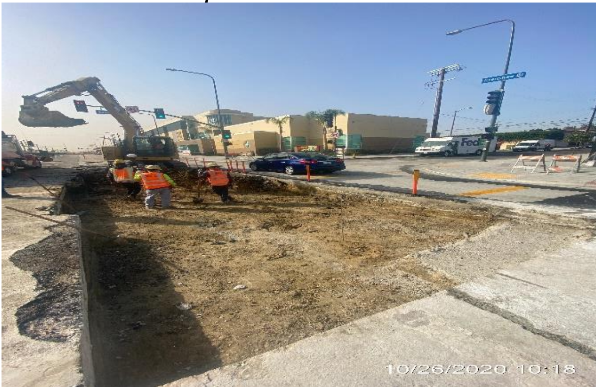
PARK MESA – Excavating existing roadway slab and setting elevations on southbound Crenshaw Blvd and 52nd St.
