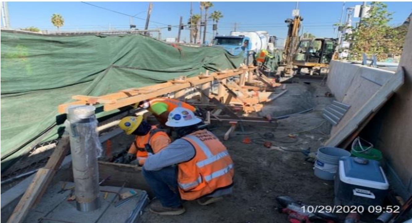
EXPO STATION – Continue setting and building formwork for the west side bollard foundations at the plaza.
