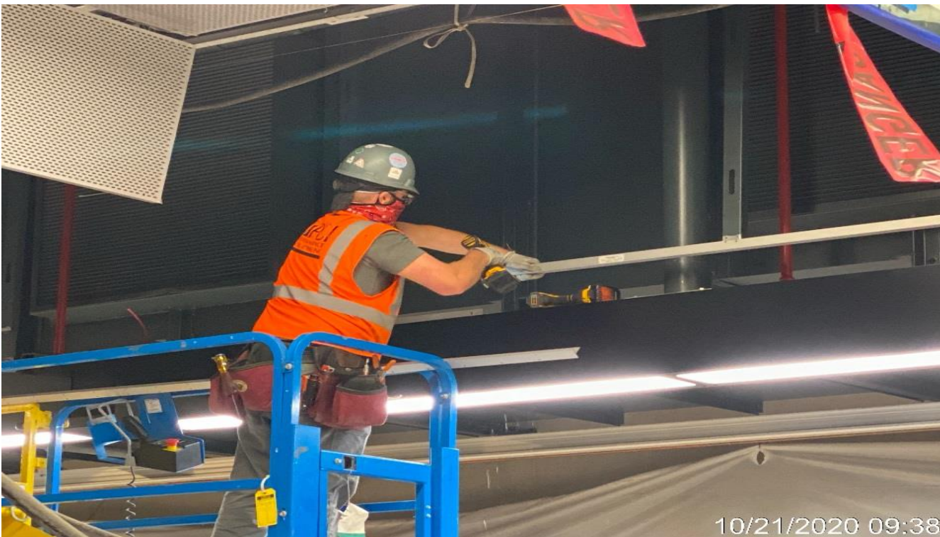
LEIMERT PARK STATION – Installing diagonal screen ceiling panels on the NB side of the platform.
