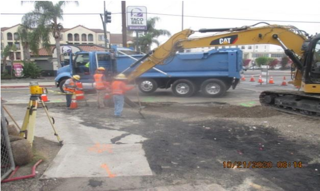
PARK MESA – Excavating northbound lane for new curb and gutter installation on the northeast corner of Crenshaw Blvd and 60th St.
