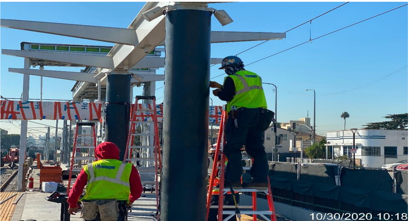
HYDE PARK STATION – Continue installing stainless steel cladding covers for the platform columns.
