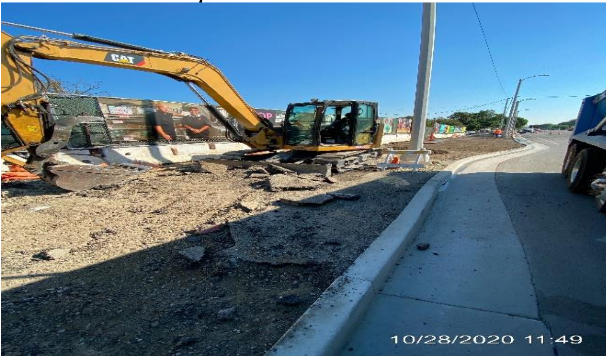
EXPO STATION – Continue excavating/grading sidewalk on westbound Obama Blvd and Crenshaw Blvd.
