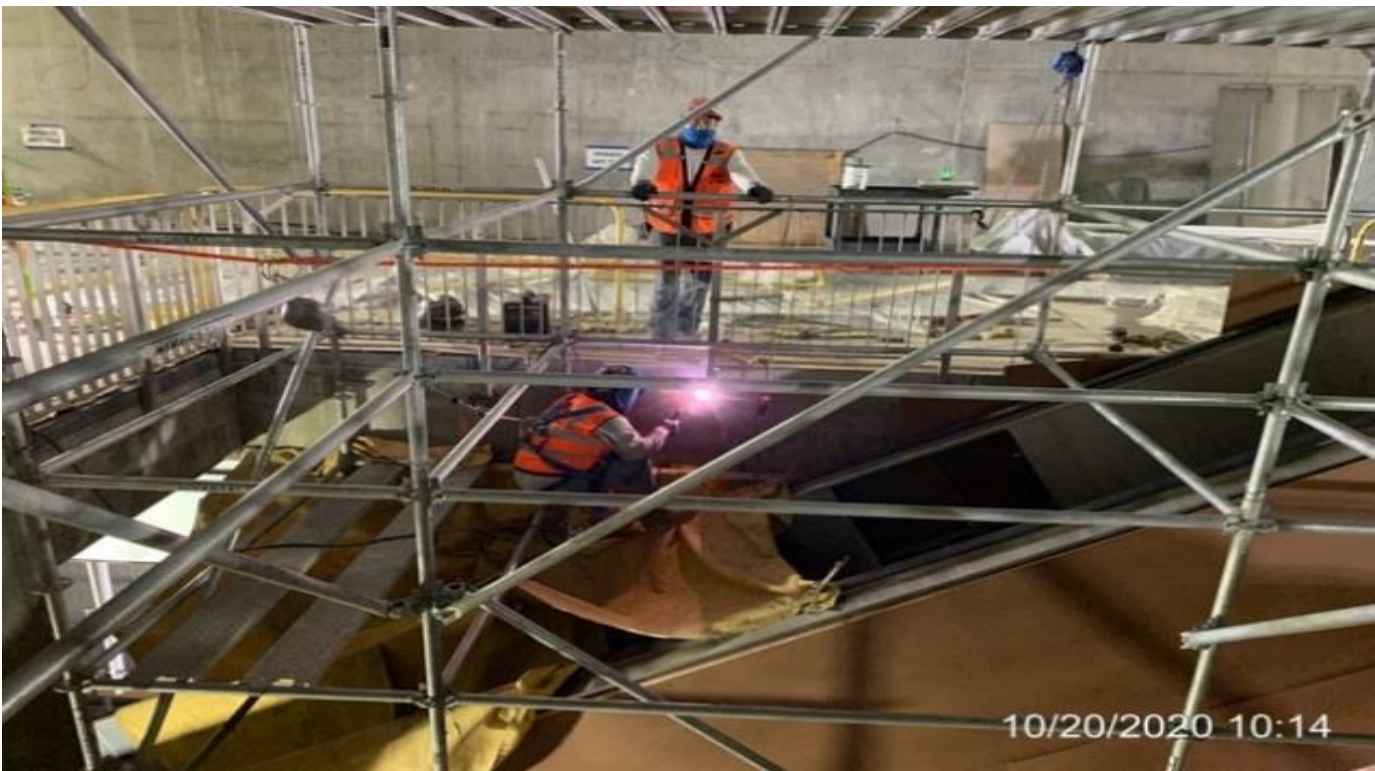
EXPO STATION – Installing/welding guardrails around the perimeter top floor opening leading into the platform and Staircase 3.
