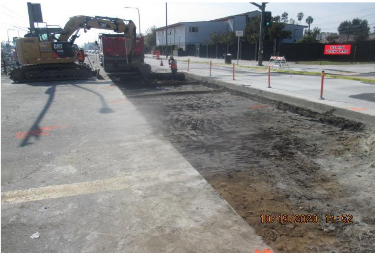
PARK MESA – Removed road slab on southbound Crenshaw Blvd and 57th St.
