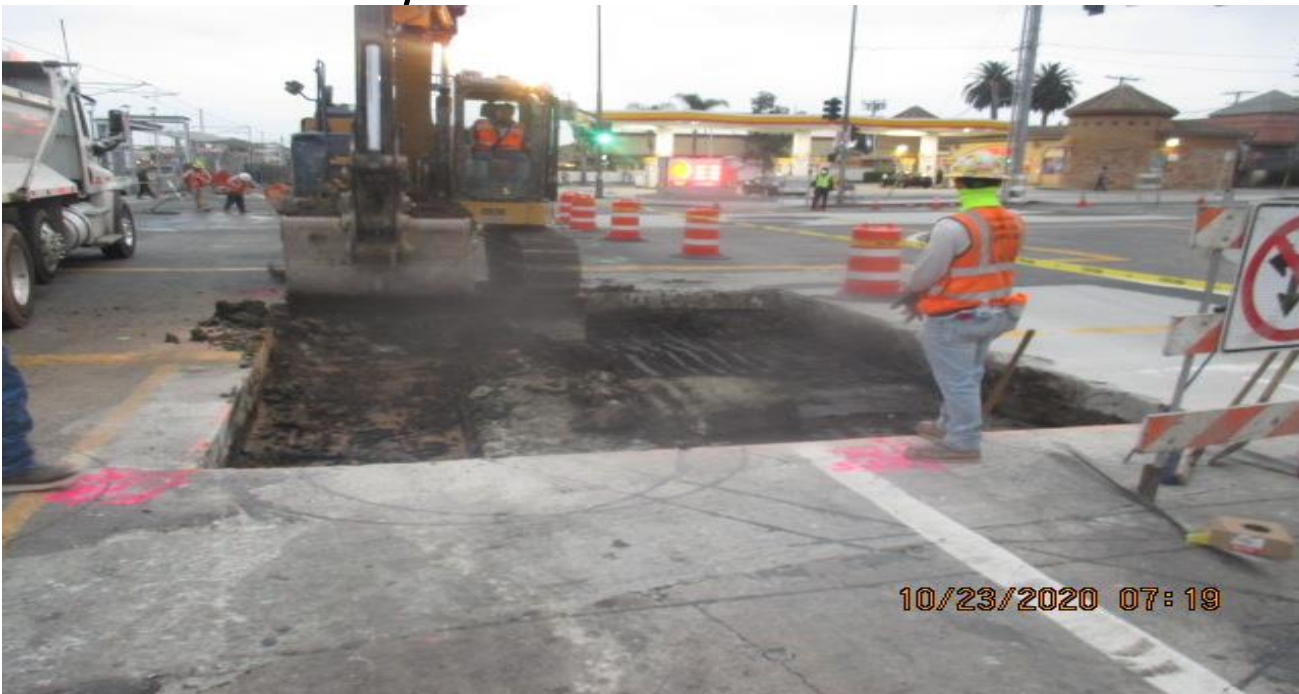
PARK MESA – Saw cut and excavated concrete slabs on the intersection of Crenshaw Blvd and Slauson Ave.
