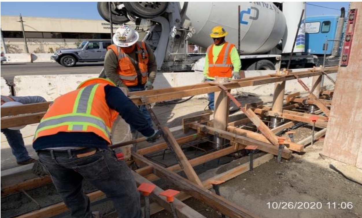
EXPO STATION – Placing concrete for the west side bollard foundations at the plaza.
