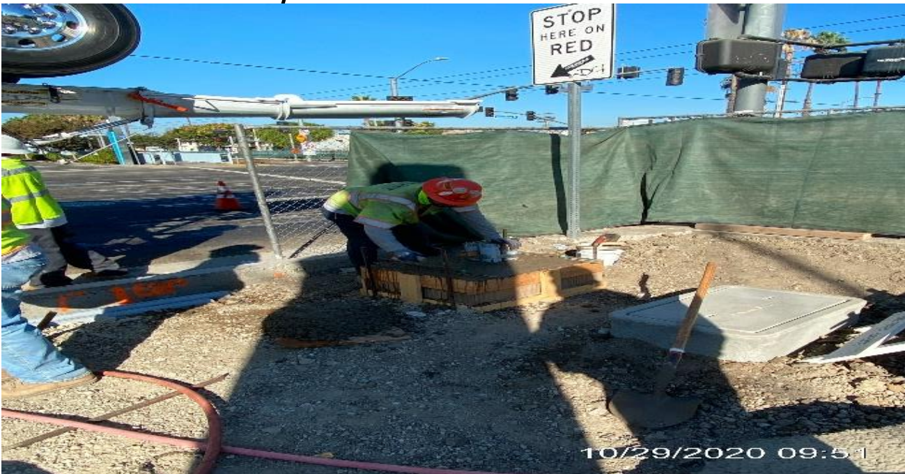
EXPO STATION – Placing concrete for traffic signal pole foundation on southeast corner of Crenshaw Blvd and Exposition Blvd.
