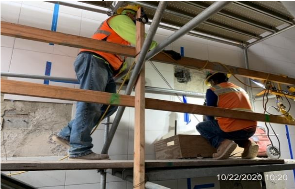
EXPO STATION – WSCC finishers removing tile and drilling into wall to expose conduit.
