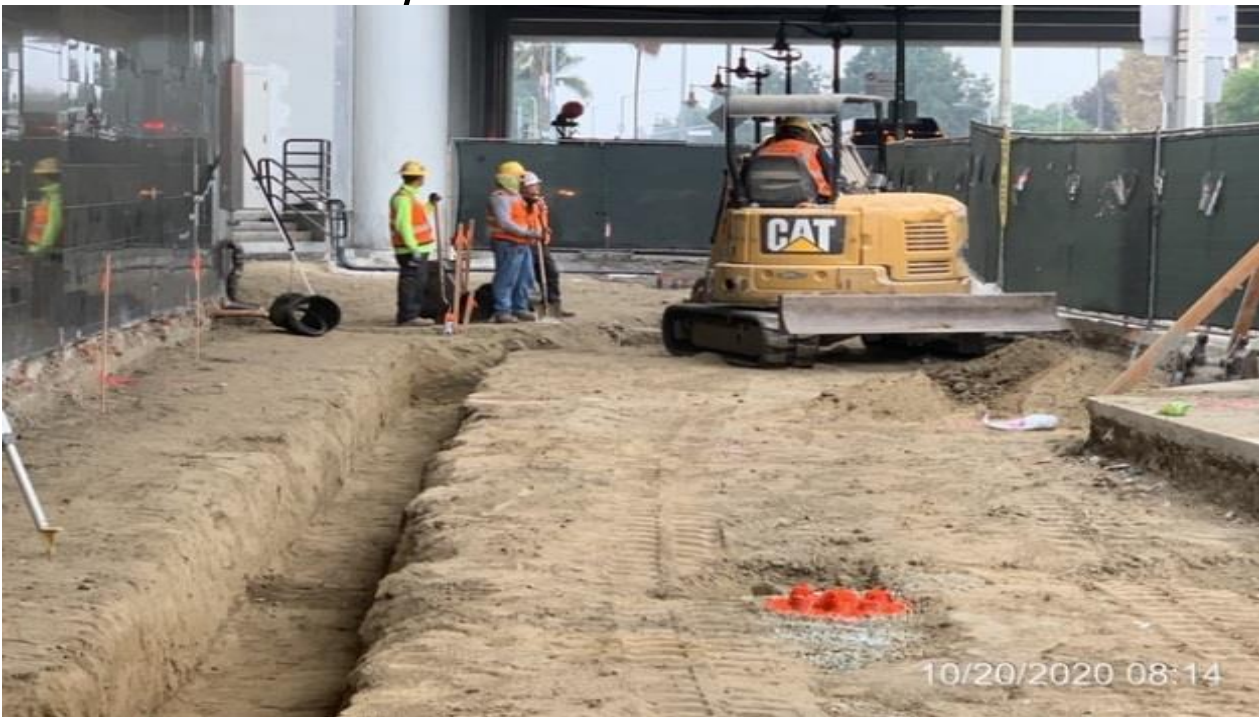
MLK STATION – Excavating/trenching for mall roof drainage at the far northwest area of the plaza.
