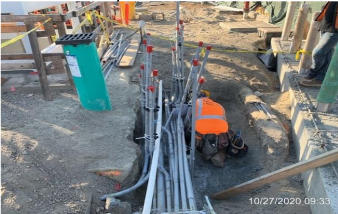
EXPO STATION– WSCC carpenters building formwork for bulk heads for conduit runs.
