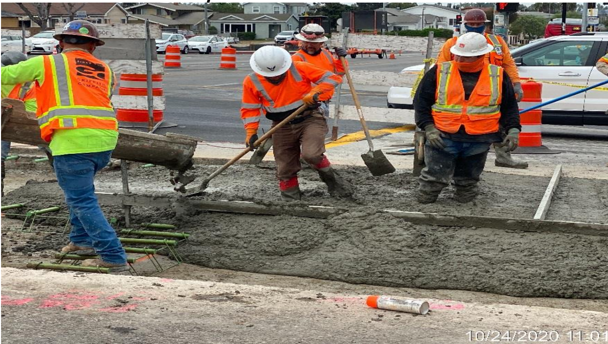
PARK MESA – Continue placing concrete slurry for roadway panels on northbound Crenshaw Blvd and Slauson Ave.
