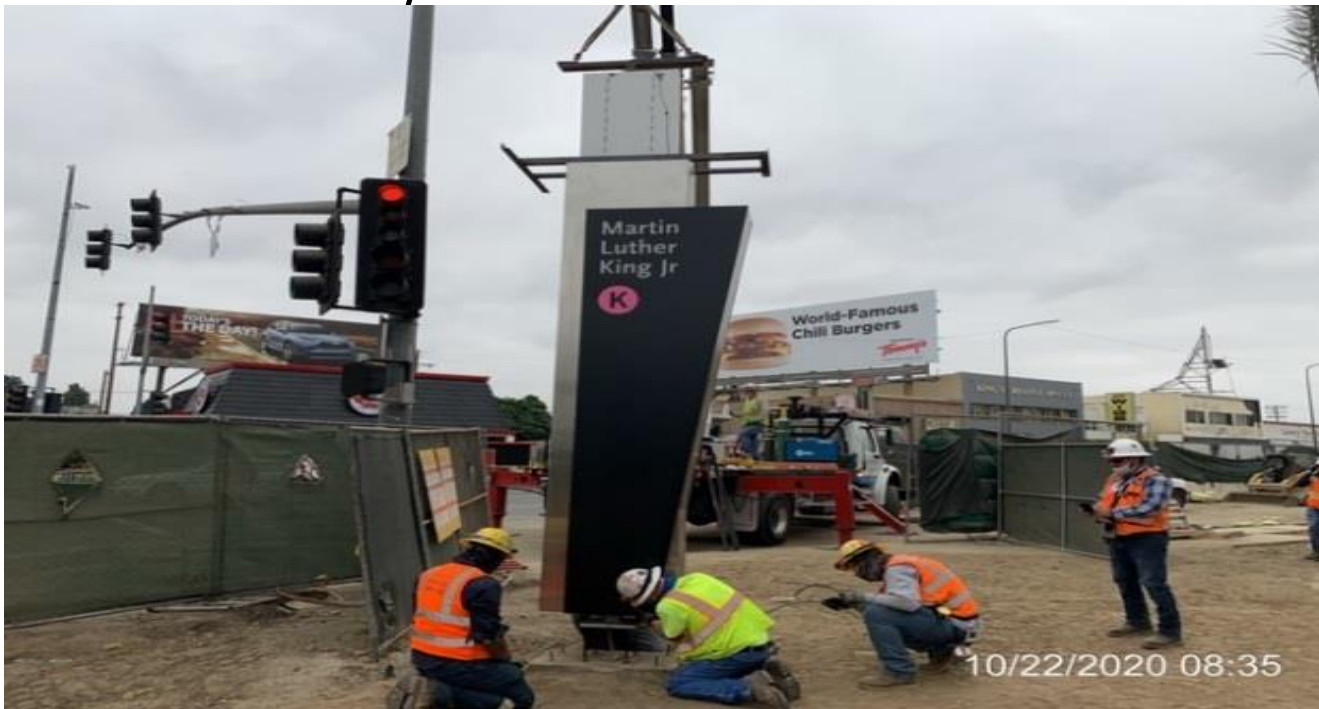
MLK STATION – Installing the Grand Pylon sign at the northeast corner of the plaza.
