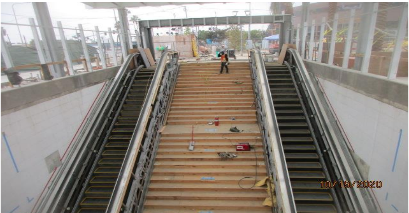
EXPO STATION – Continue installing brackets for handrail installation for Staircase 1 at the main entrance.
