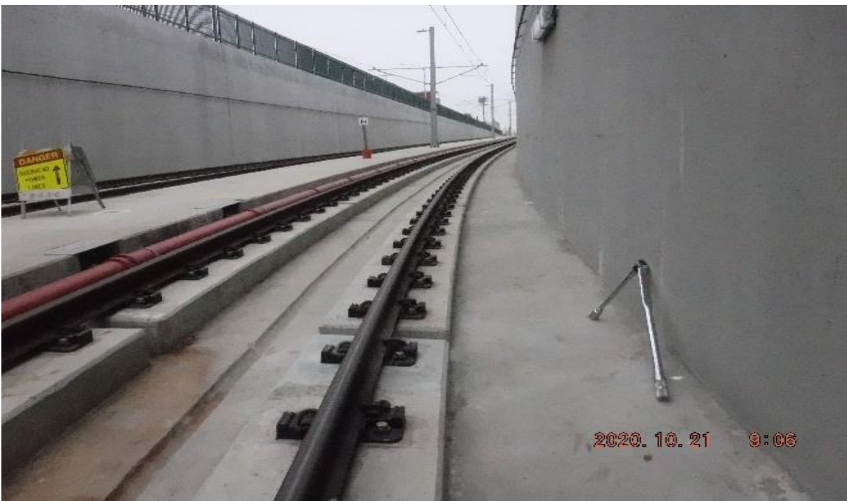
UG3 – STA 284+00 TK#4/NB looking south – DF's AB torque in UG3 – Victoria (REWORK)
