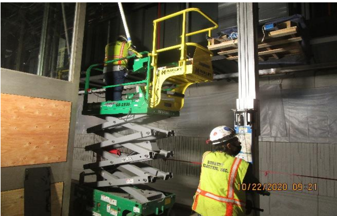
MLK STATION – MLK North platform resume installing Edge lighting fixtures at reworked edge lighting support posts.
