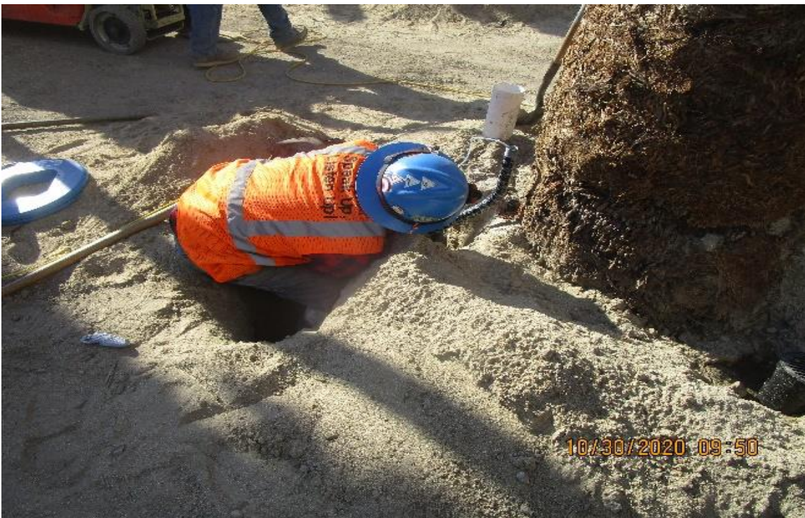
MLK STATION – MLK South Plaza, Begin Reworking 1” GRC landscape lighting to allow grate clearance & installation.
