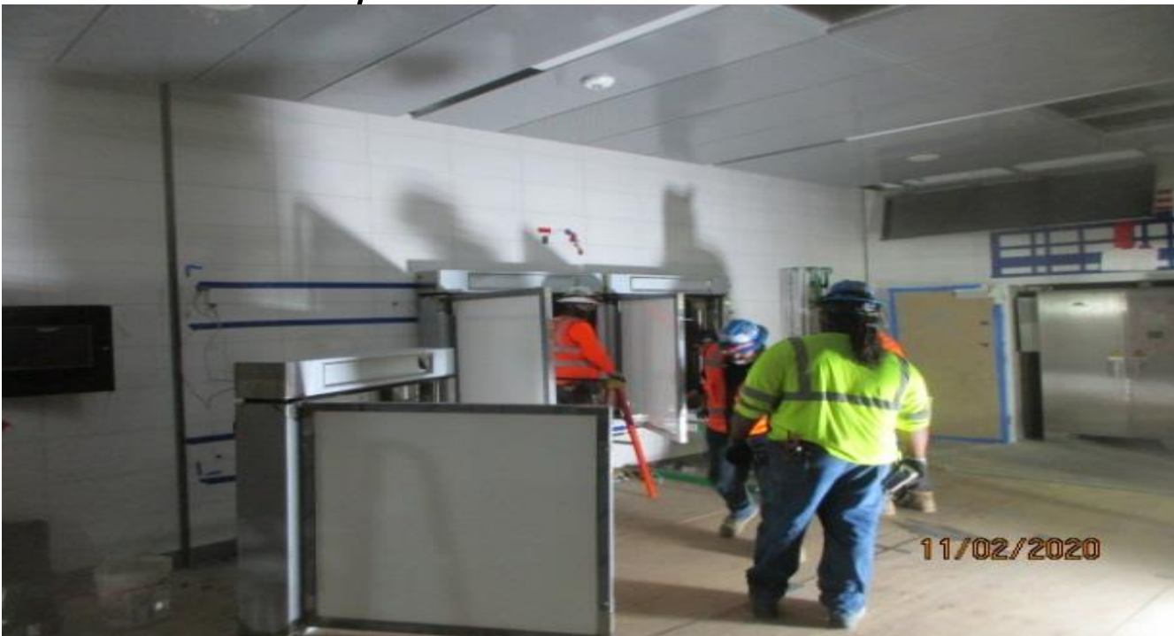
EXPO STATION – Installing map case on the east wall of the Paid Area at the concourse.
