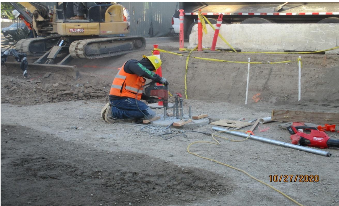
AVIATION/CENTURY- Chipping out the anchor bolts on the light pole foundation at the Aviation Station due to an incorrect bol.
