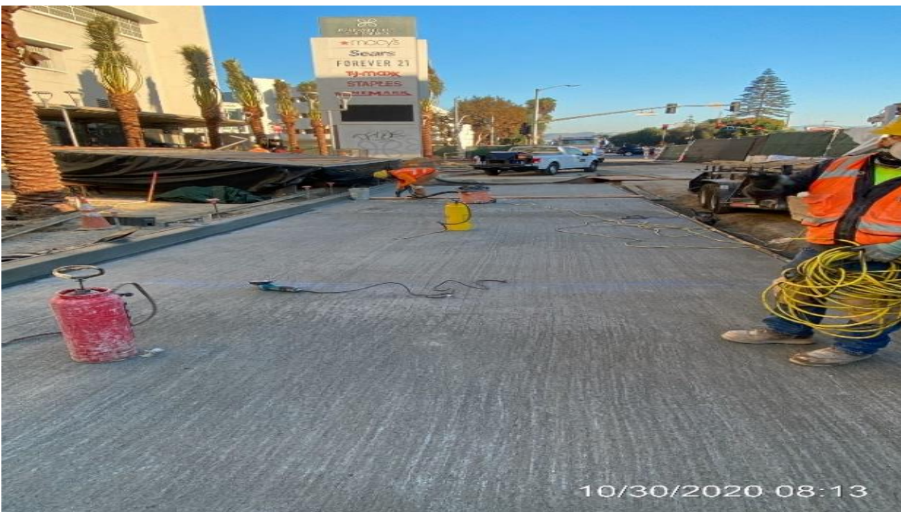
MLK STATION – Removing formwork and saw-cutting curb/gutter and bus pad bay along the east side of the plaza.
