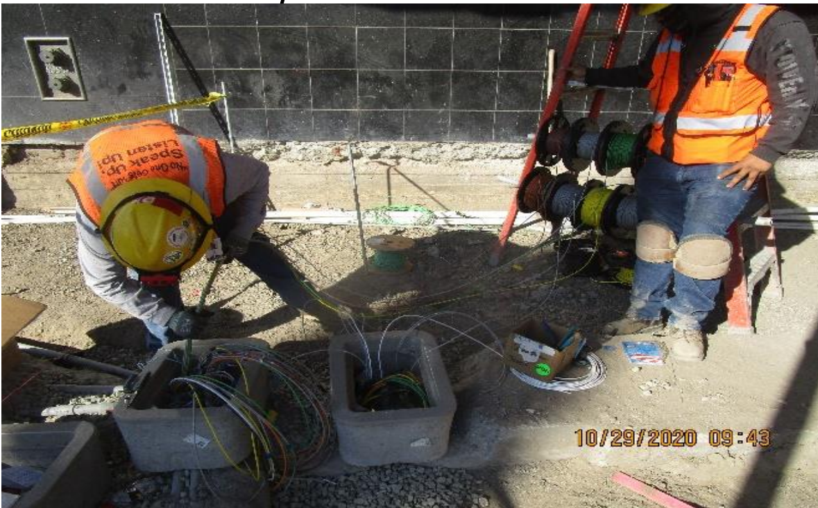
MLK STATION – MLK Plaza, (N) continued Pulling #10 XHHW-2 lighting wiring & setting embedded pull boxes to finish elevation.
