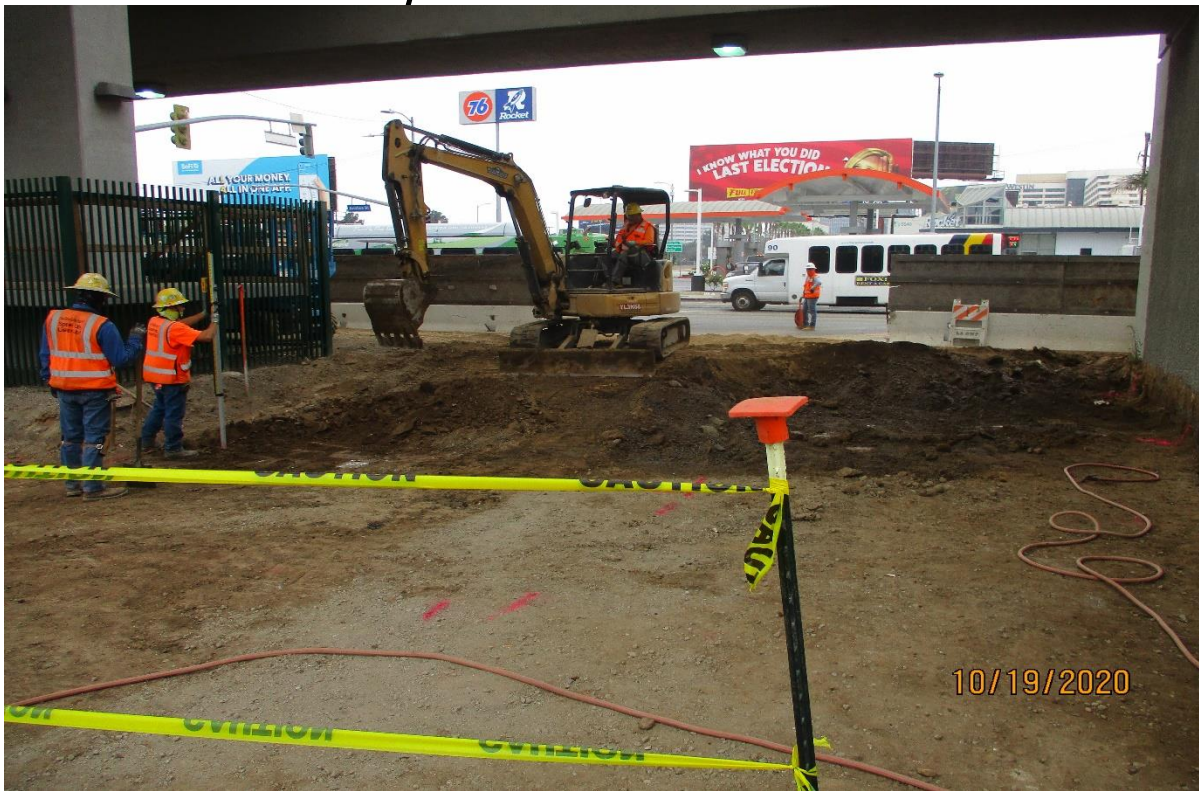
AVIATION/CENTURY- Excavating for the amended soil at the Sw corner of Aviation and Century.
