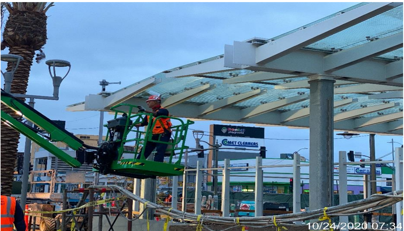
EXPO STATION – Drilling holes to the main entrance canopy structure for BOCA lighting at the plaza.
