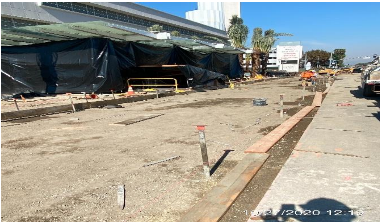
MLK STATION – Setting elevations and placing formwork along the east side of the plaza for new curb/gutter and bus pad installation.
