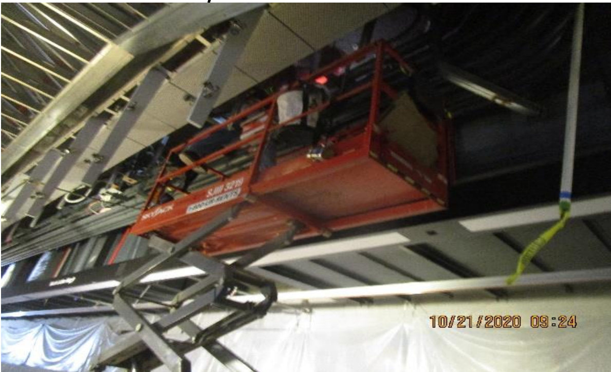
MLK STATION – MLK Platform, NB & SB tracks, continued piping 1" GRC & ¾" seal tight (speaker & FA) to edge lighting.
