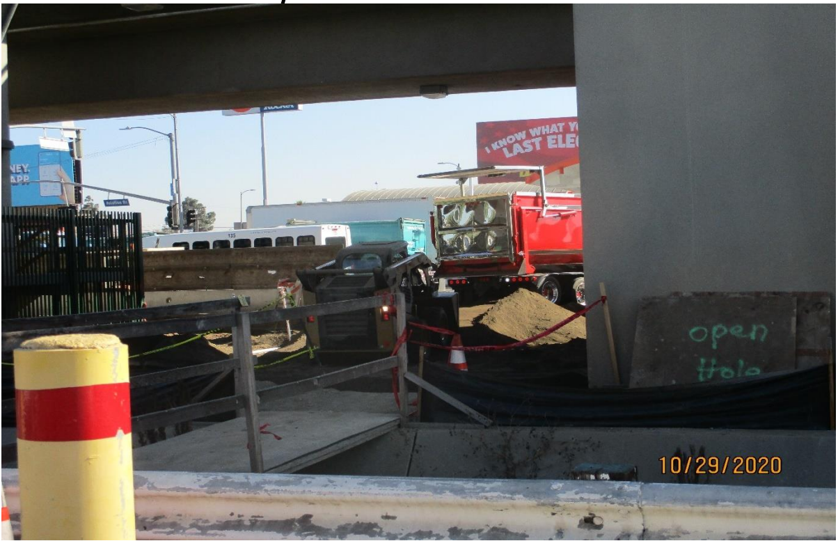
AVIATION/CENTURY- Placing amended soil on the Sw corner of Aviation and Century
