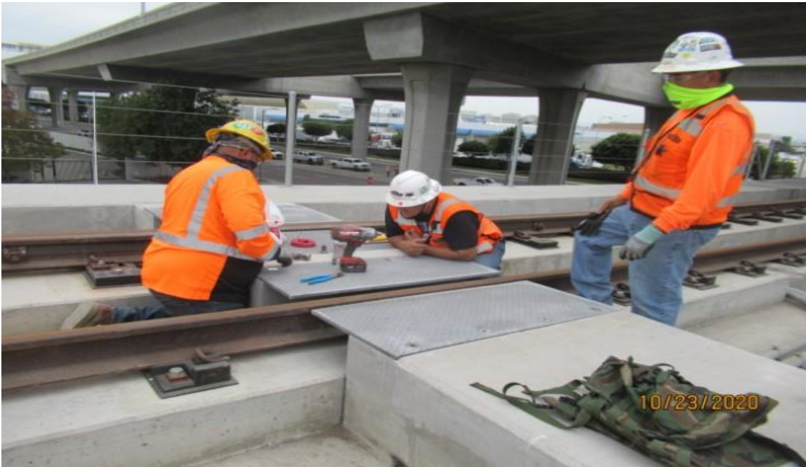
Guideway- WSCC at west leg of Wye SBW STA 13+52 re-placing damaged emergency walkway plate bolts (looking northwest) Rework
