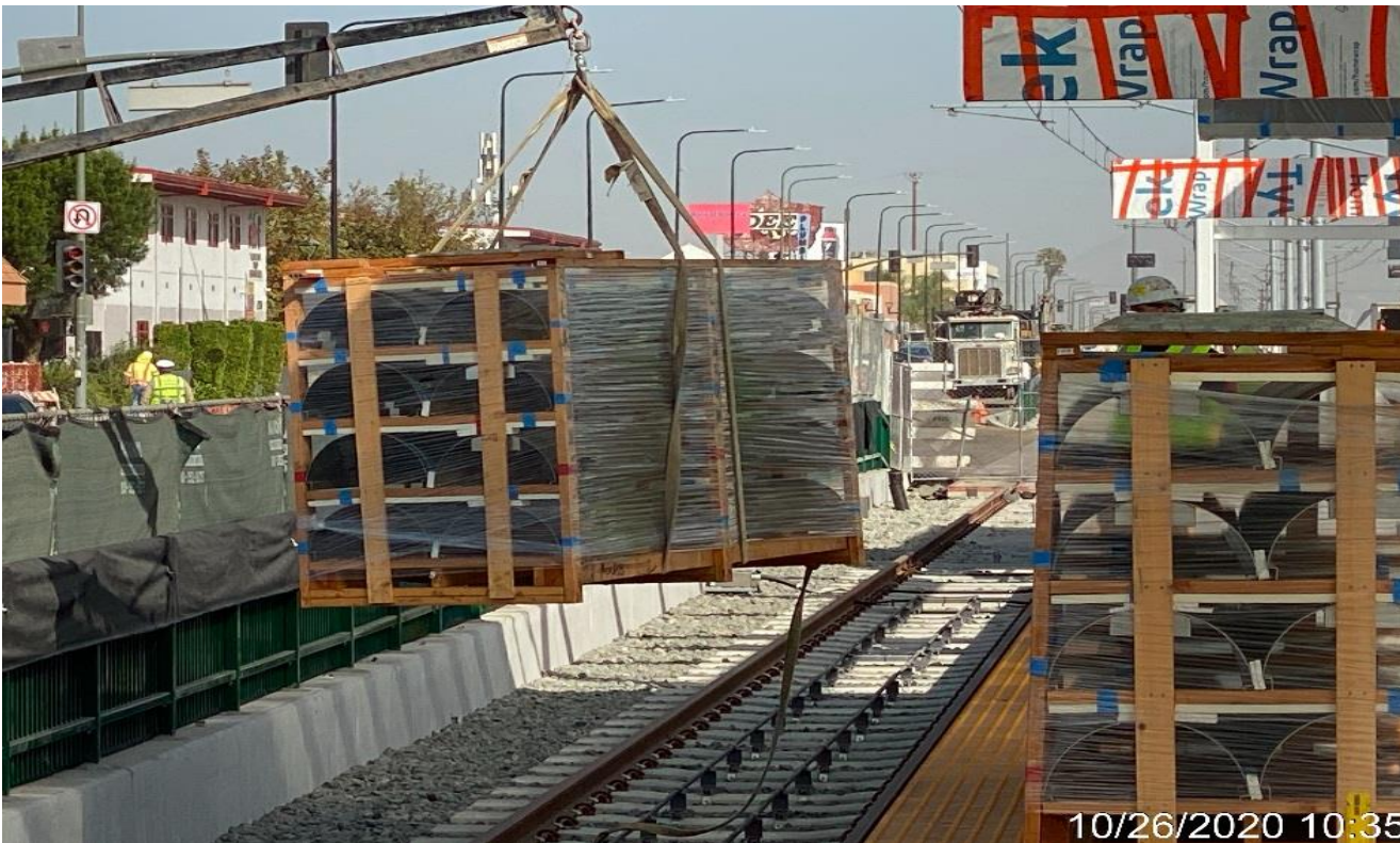
HYDE PARK STATION – Delivering stainless steel cladding for the platform columns covers.
