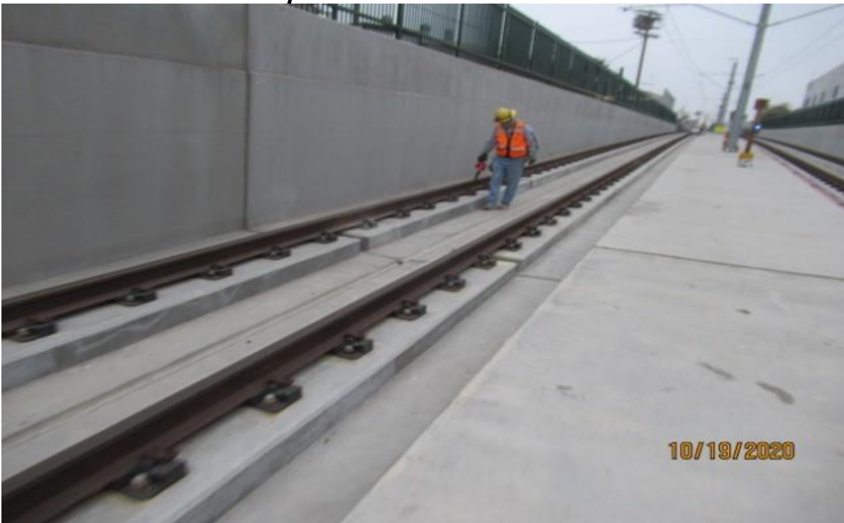
UG3 – WSCC preparing to butter top of plinths south end UG3 (looking south).
