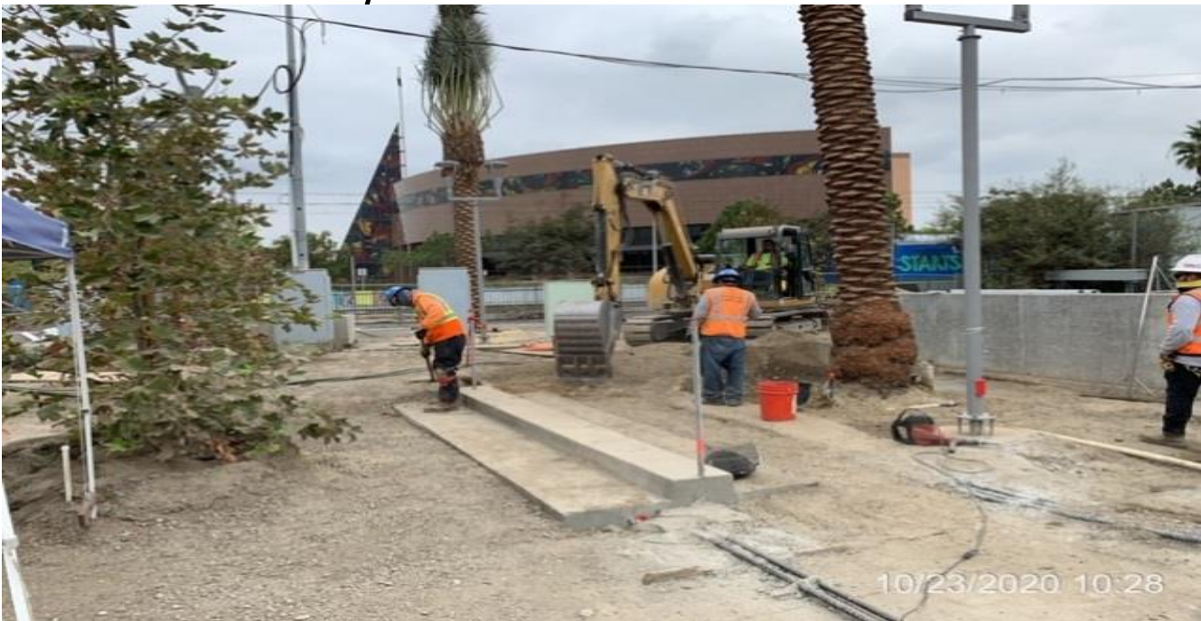
EXPO STATION – Fine grading and compacting the northwest area of the plaza.
