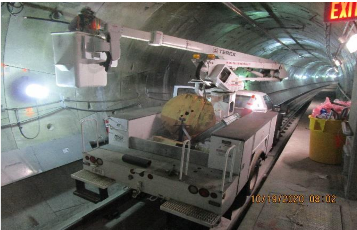
MLK STATION – Southbound bored tunnel Vernon to MLK Begin removing 1-1.4” Radiacx cable between CP5 & (S) MLK portal
