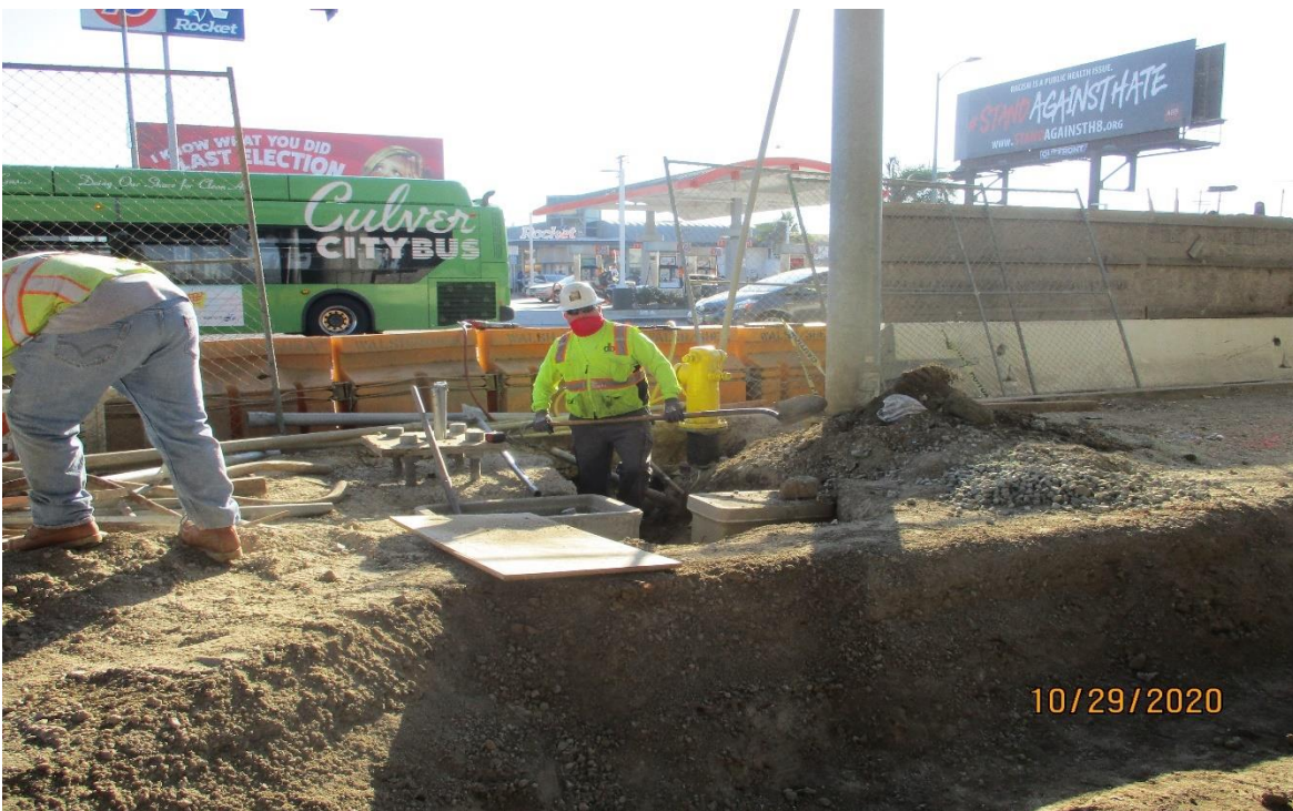
AVIATION/CENTURY- Traffic signal conduit installation for the Sw corner of Aviation and Century.
