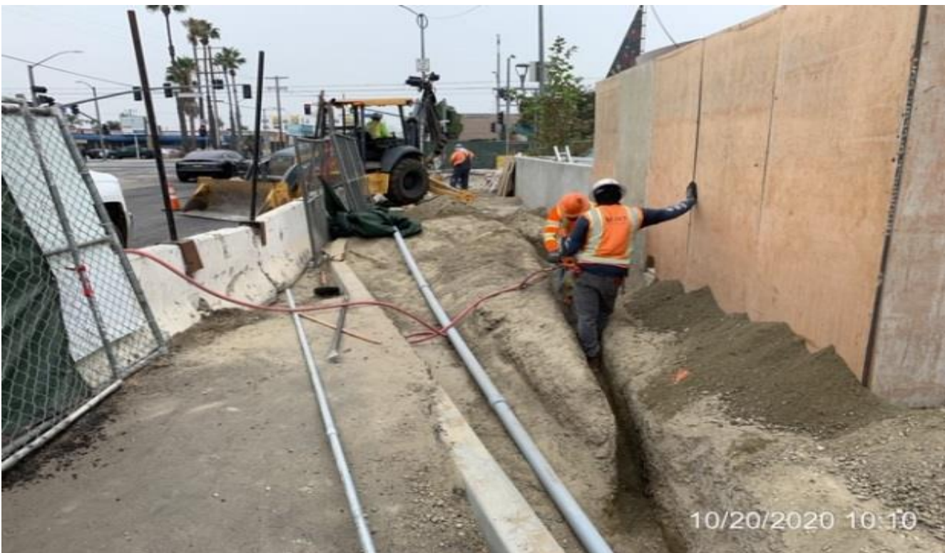
EXPO STATION – Excavating/trenching to extend conduit for landscape lighting at the northwest area of the plaza.
