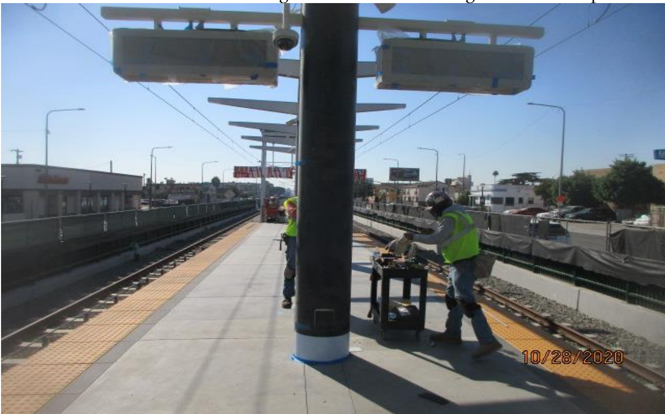
HYDE PARK STATION – Continue installing stainless steel cladding covers for the platform columns.
