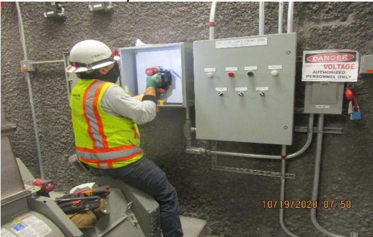
Crenshaw/Vernon – Vernon, Mechanical (S) C114, begin rough in 480,120 Sola HD transformer between disconnect & ACCP-1.
