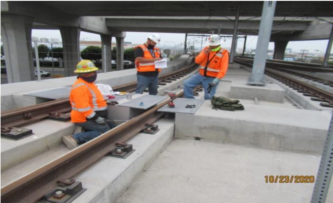
Guideway- WSCC at west leg of Wye SBW STA 13+52 re-placing damaged emergency walkway plate bolts (looking north) Rework
