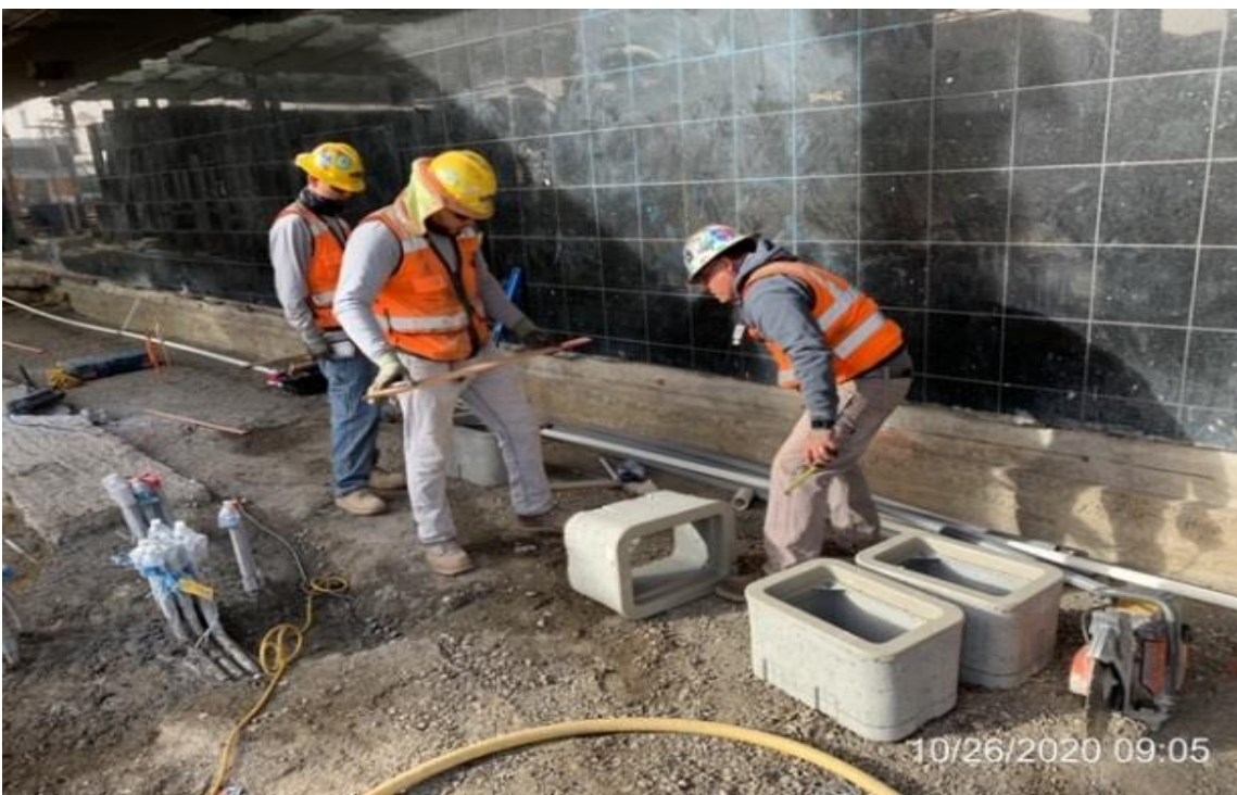
MLK STATION – WSCC crew chipping concrete encasement and modifying concrete pull boxes.
