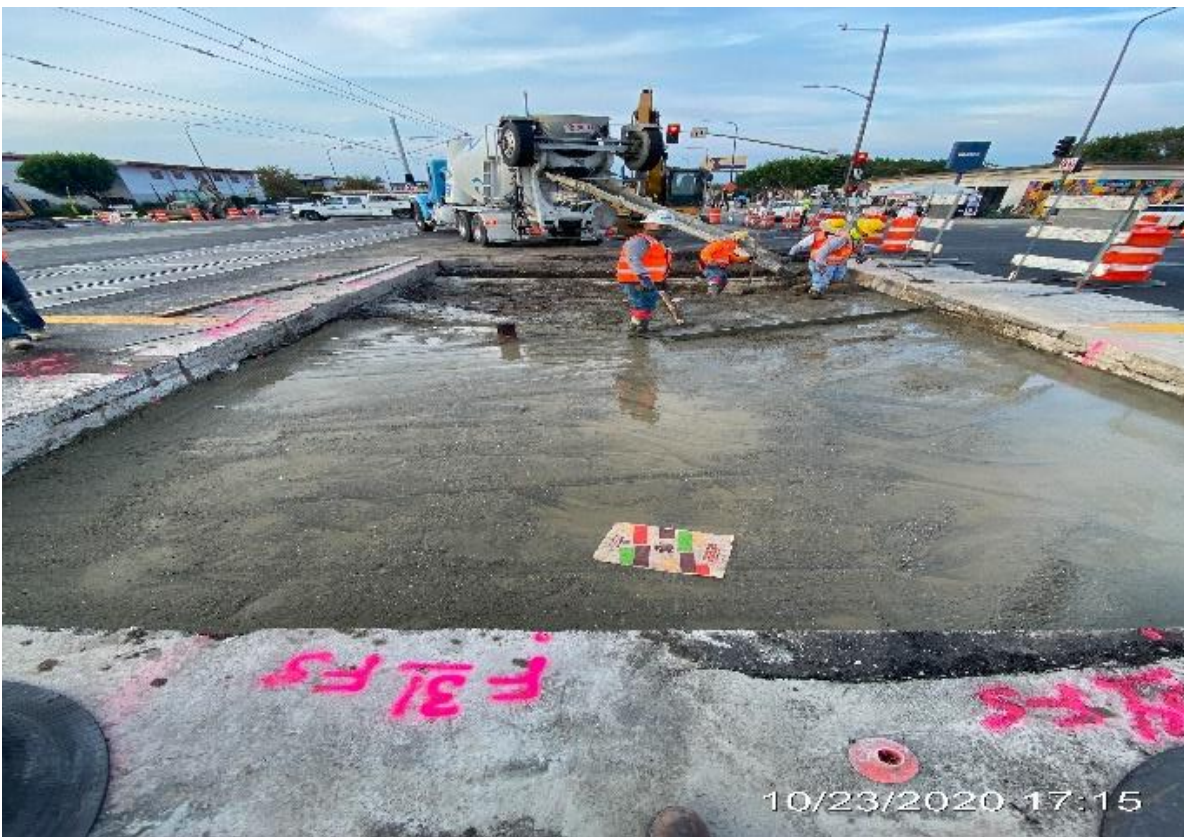
PARK MESA – Continue building formwork and placing slurry on the north and southbound lanes for restoration at the intersection of Crenshaw Blvd and 57th St.
