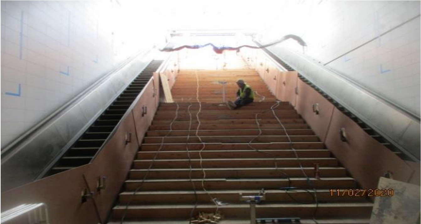
MLK STATION – Continue layout and coring of Staircase #1 for handrail installation from plaza to concourse.
