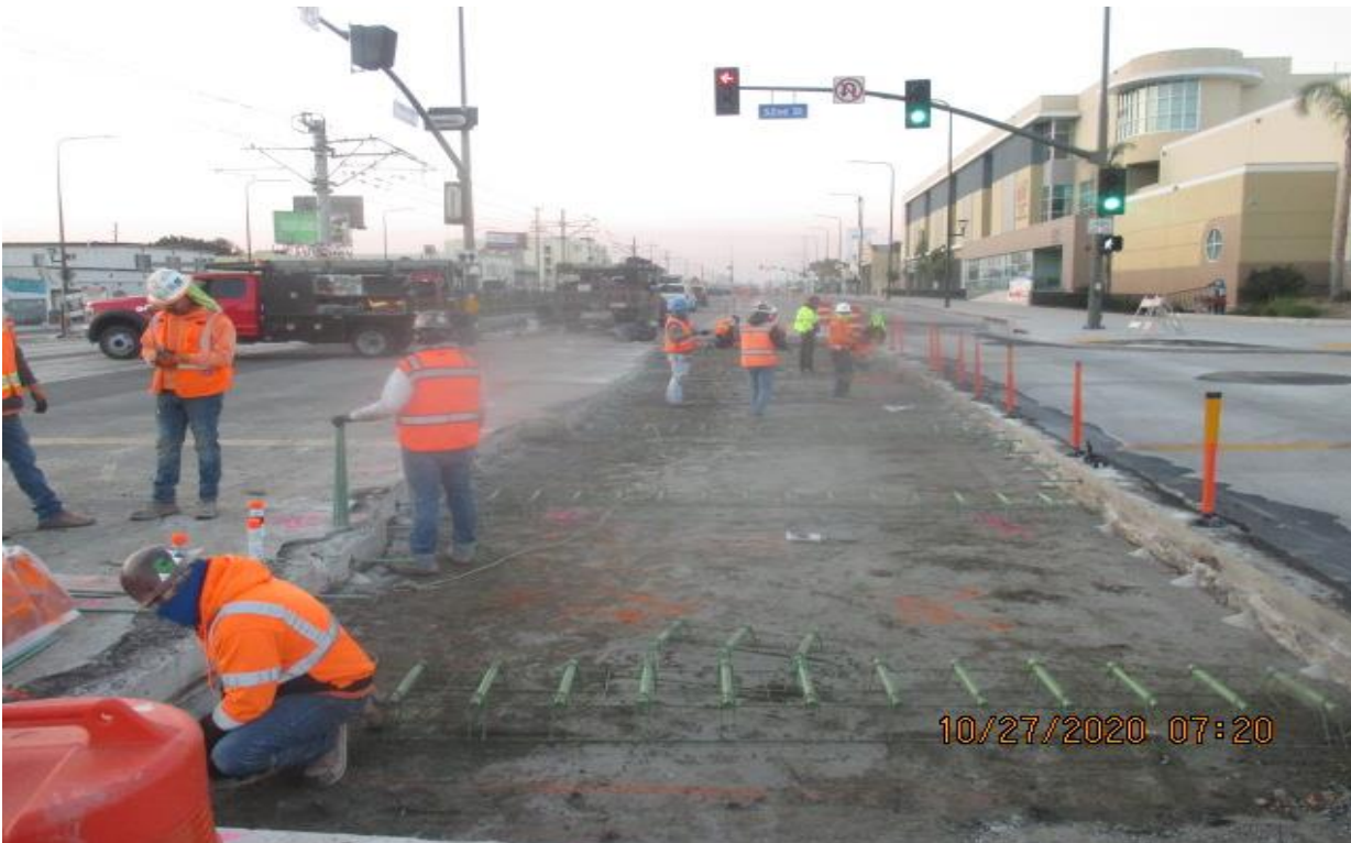
PARK MESA – Placing rebar in preparation for concrete placement of the existing roadway slab on southbound Crenshaw Blvd and 52nd St.
