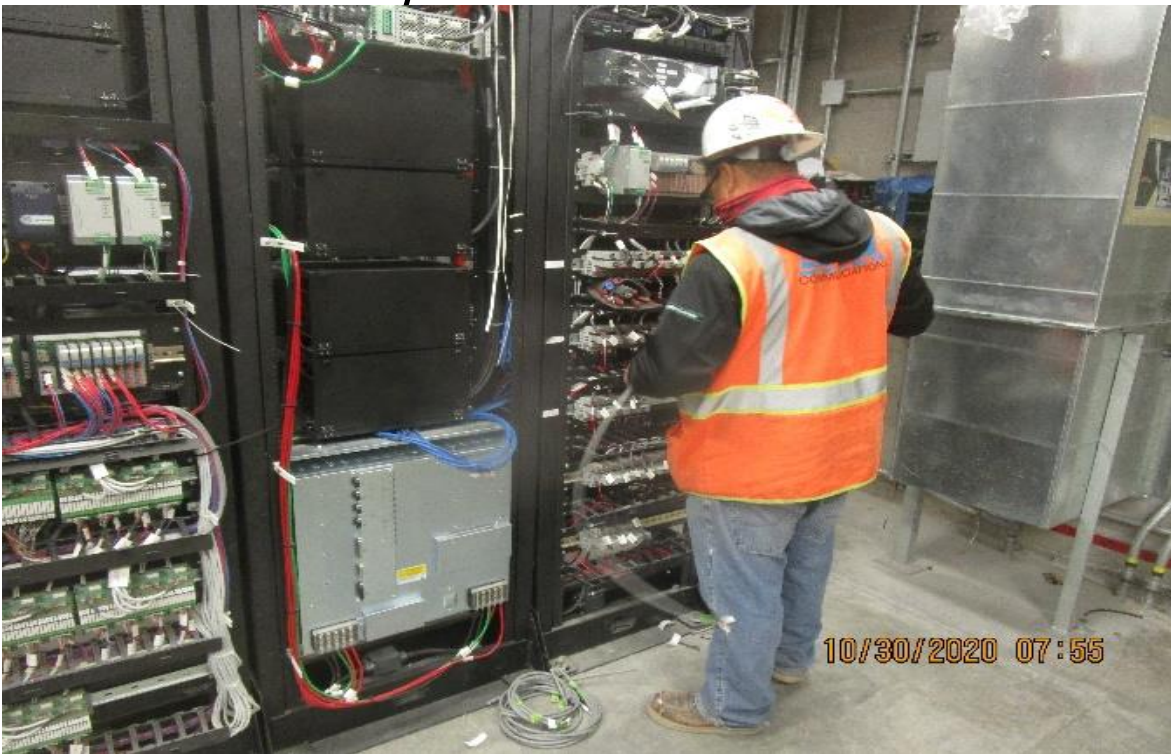
Crenshaw/Vernon – Vernon Concourse, TC&C Room C112, Resume SCADA terminations 5 pair #22`s (seismic gas sensors) at MDF-1
