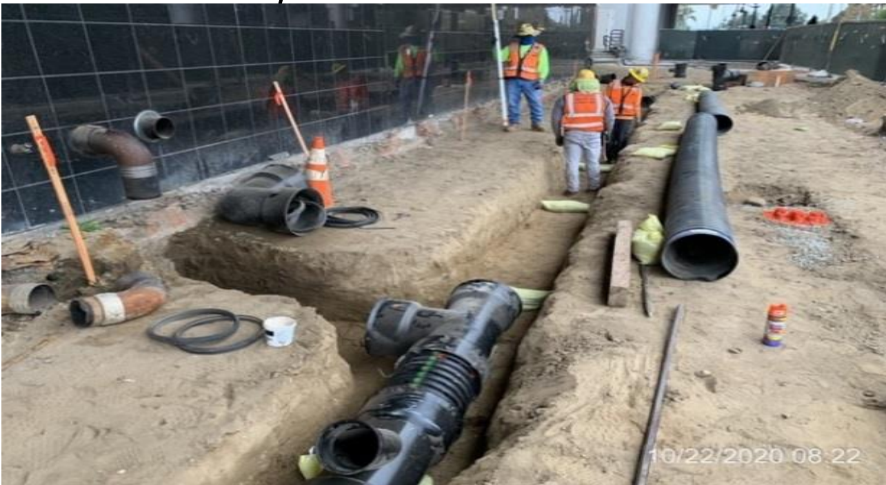
MLK STATION – Continue laying down HDPE pipe for the mall roof drainage at the far northwest area of the plaza.
