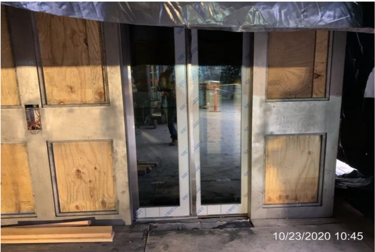
EXPO STATION – Broken exterior glass pane (right side) at platform, elevator #1.
