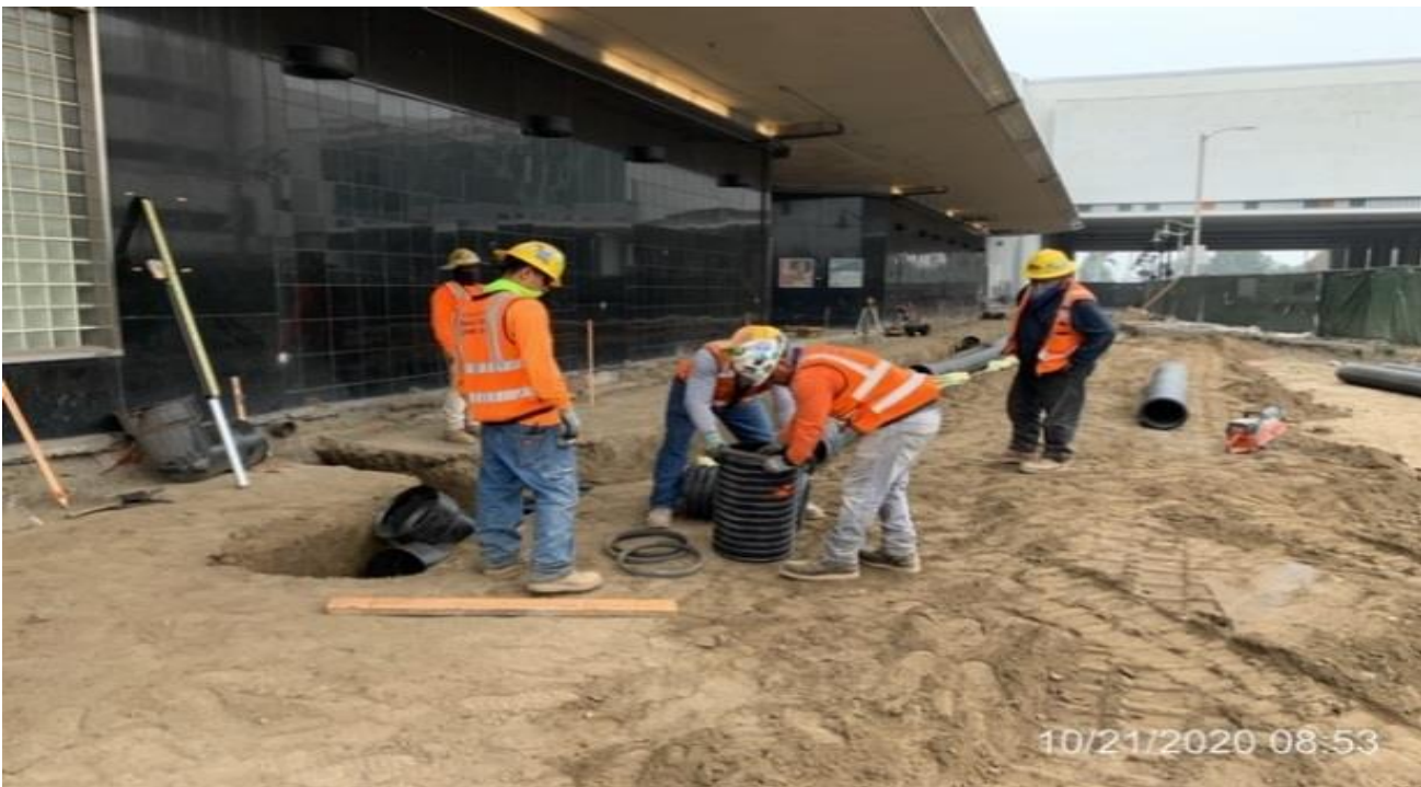
MLK STATION – Laying down HDPE pipe for the mall roof drainage at the far northwest area of the plaza.
