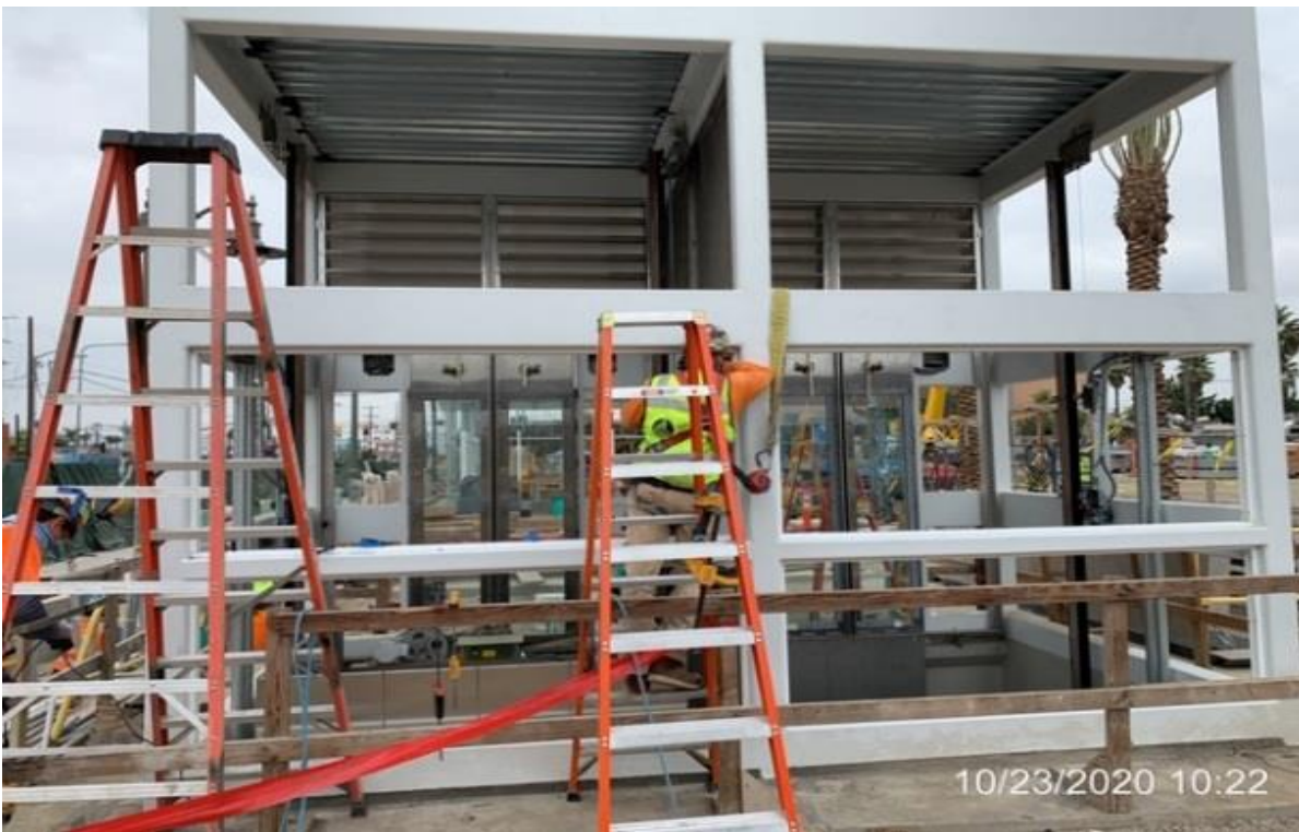
EXPO STATION– Giroux Glass fabricating and installing glass stops for elevator structure #1 & #2
