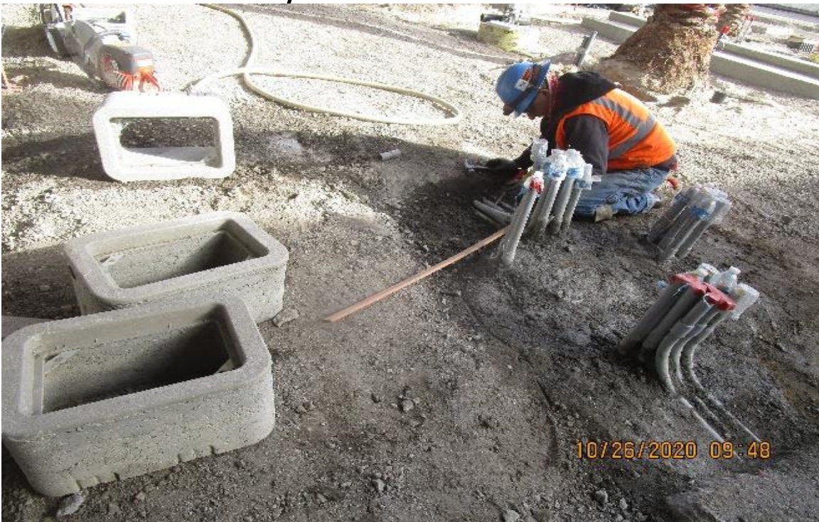
MLK STATION – MLK, (N) Plaza, begin chipping out lighting PVC conduit to lower & set embedded pull boxes to finish elevation
