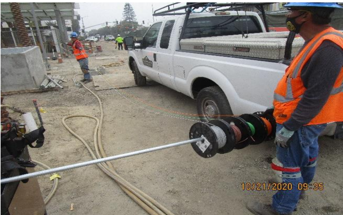
MLK STATION – MLK Plaza, North plaza continued setting embedded comm & lighting pull boxes & pulling #10 XHHW-2's.
