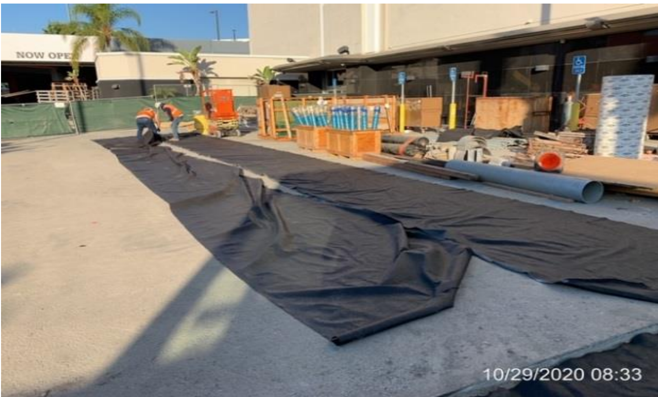
MLK STATION – Preparing to install soil liner inside the south planter wall at the plaza.
