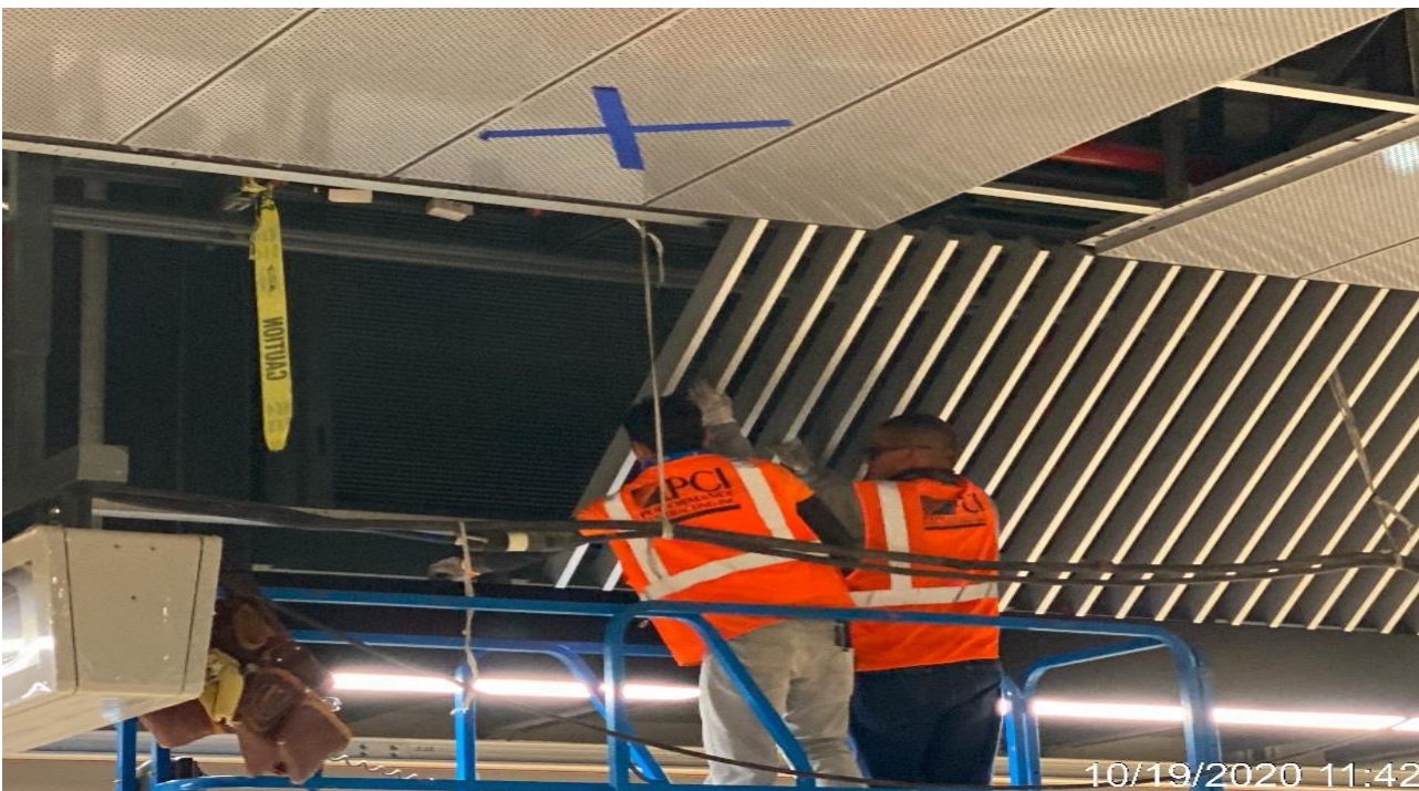
LEIMERT PARK STATION – Installing diagonal screen ceiling panels on the SB side of the platform.
