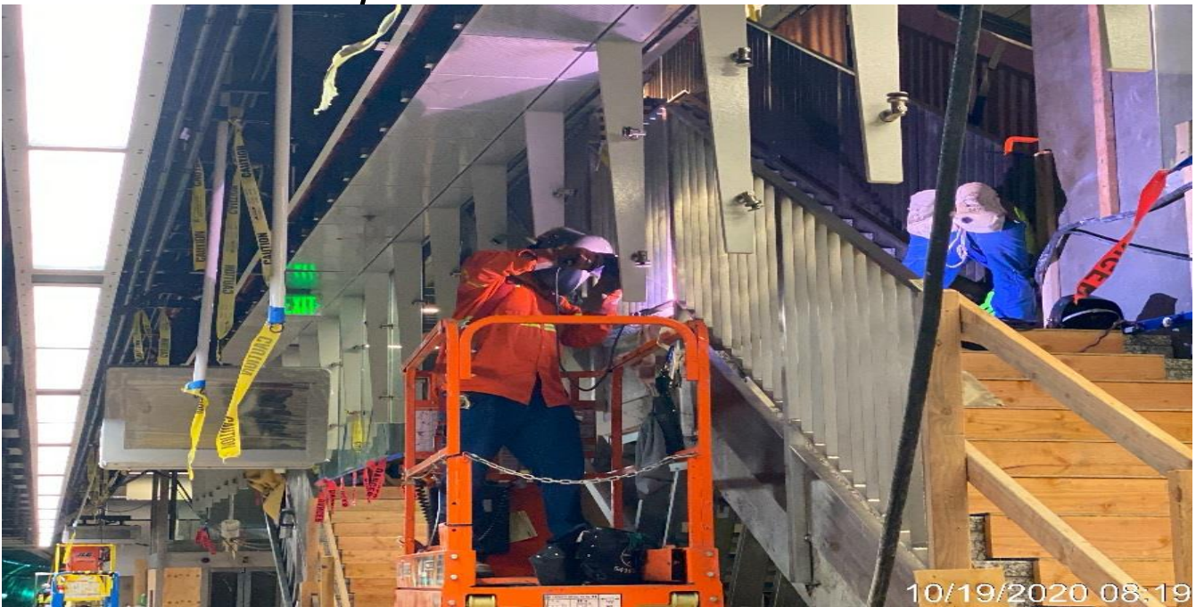
LEIMERT PARK STATION – Continue welding guardrails to Staircases 3&4 from concourse to platform.
