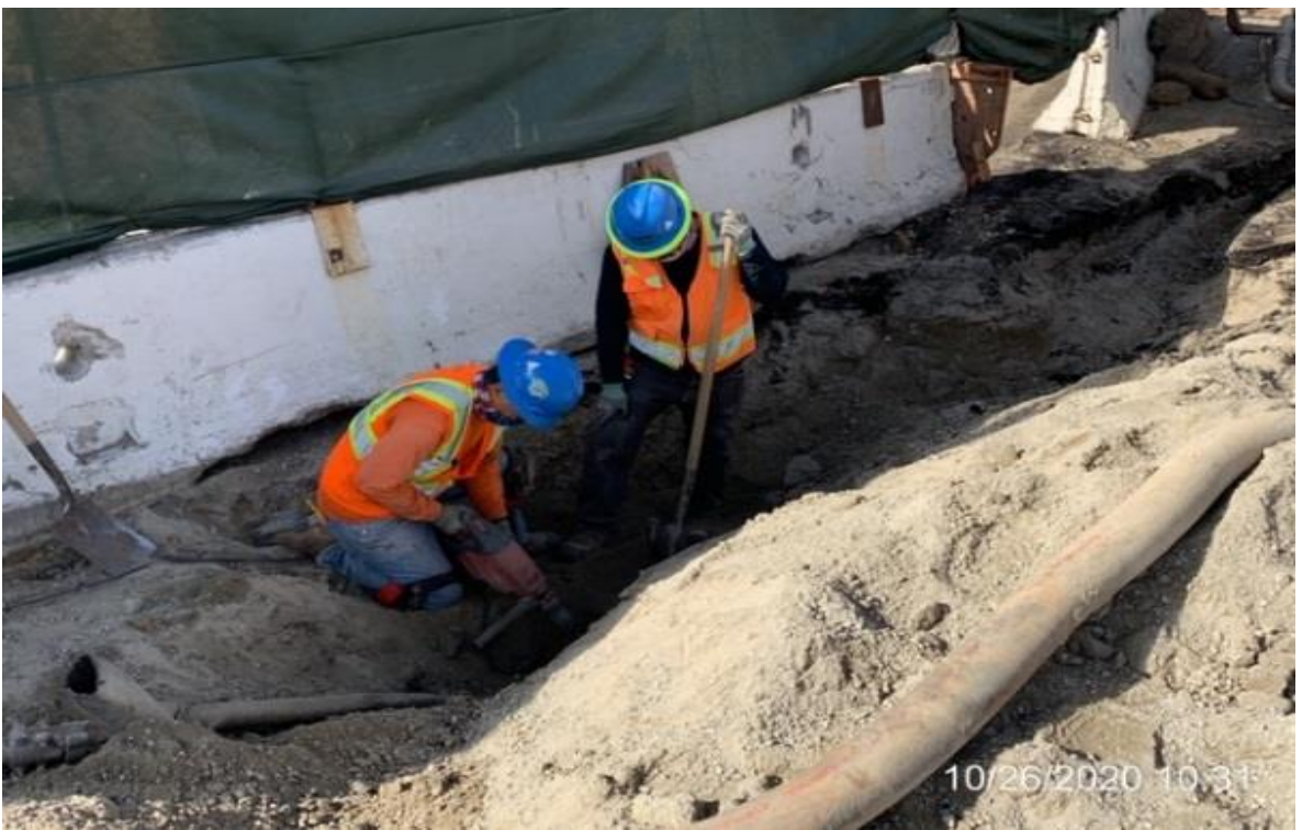
EXPO STATION – WSCC crew removing buried hoses from south side of yard prior to moving K-rail.
