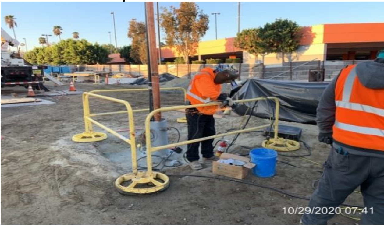
MLK STATION – Installing shaft to the south vent stack at the plaza.
