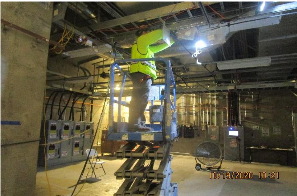
MLK STATION – MLK Invert, TPSS Room T109, Continued rework 7/8" Radiax cable separation of 8' & add supports.
