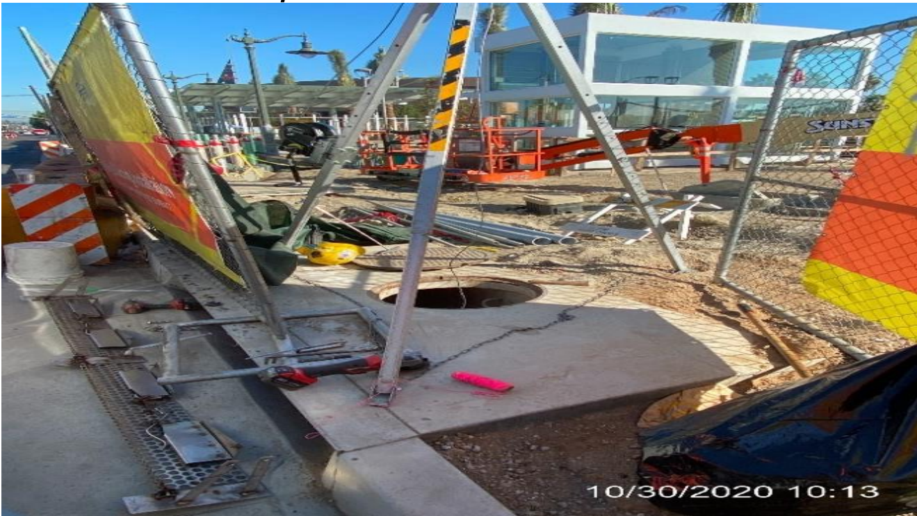
EXPO STATION – Adding screens to Catch Basin #12 on the southwest corner of the plaza.
