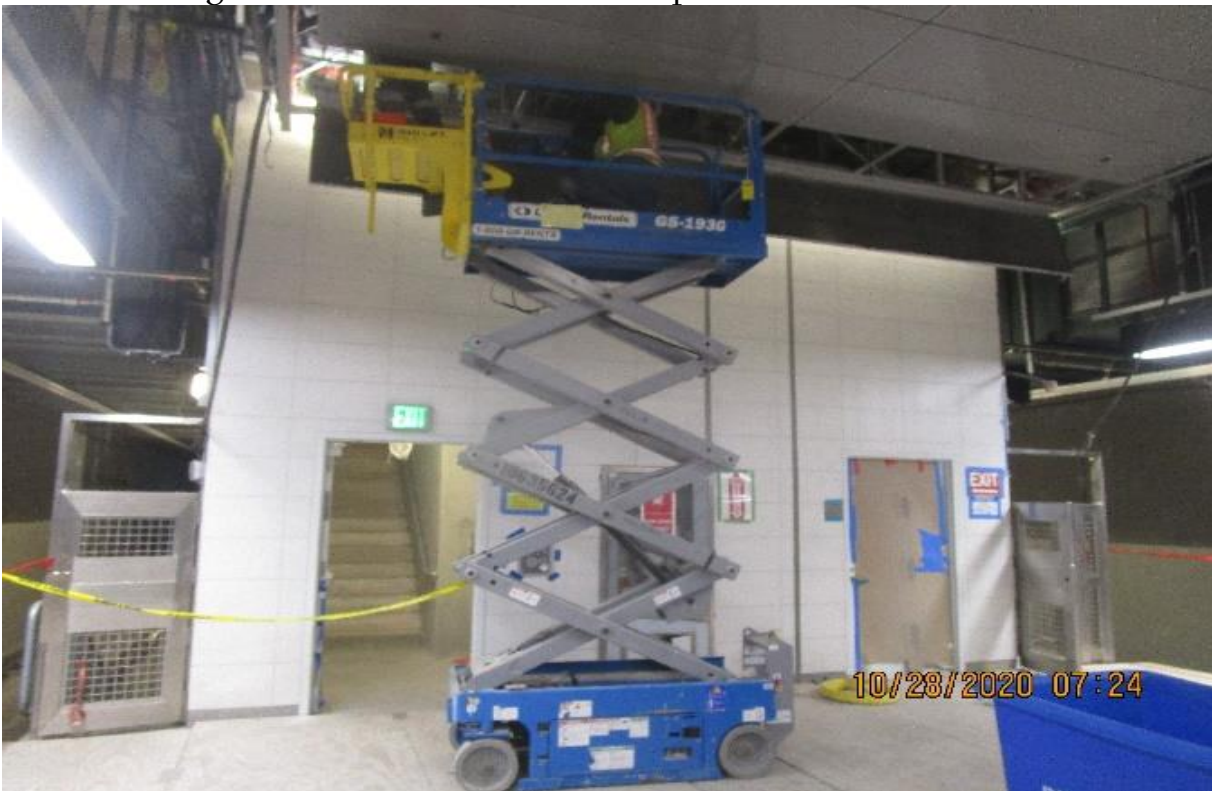
Crenshaw/Vernon – Vernon (S) Platform, continued seismic supports at 2" & 2-1/2" GRC Radiax support conduit above drop ceiling.
