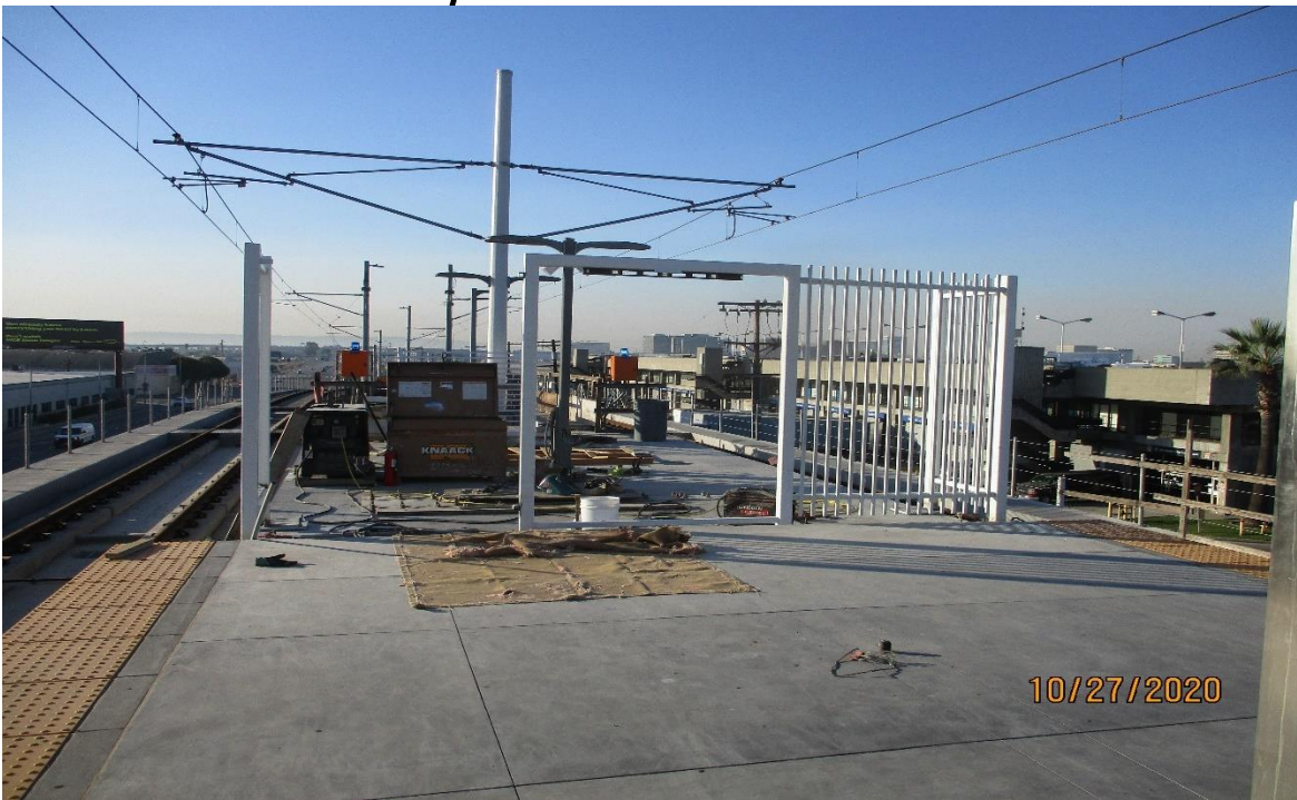
AVIATION/CENTURY- Fabrication and erection of the Aviation Station platform south emergency exit gate.
