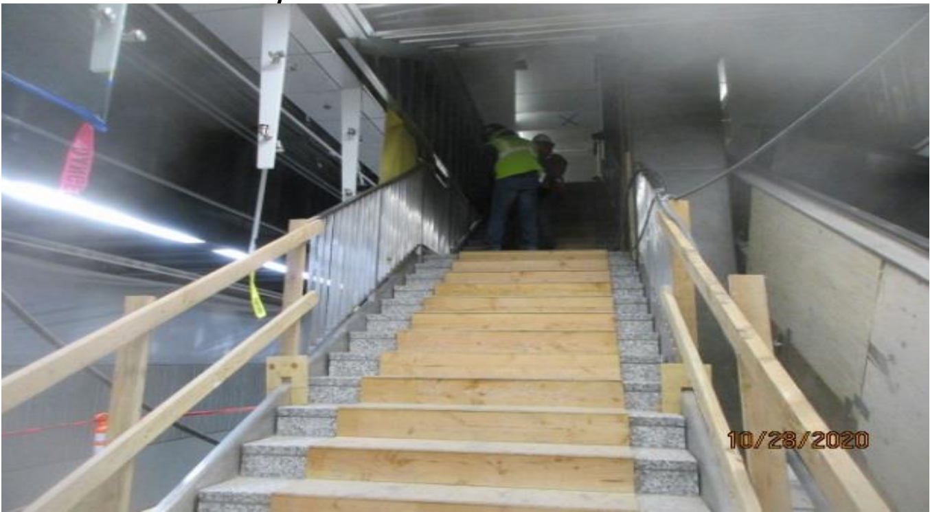
LEIMERT PARK STATION – Continue welding guardrails to Staircases 3&4 from concourse to platform.
