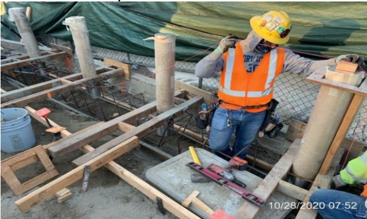
EXPO STATION – Continue setting and building formwork for the west side bollard foundations at the plaza.
