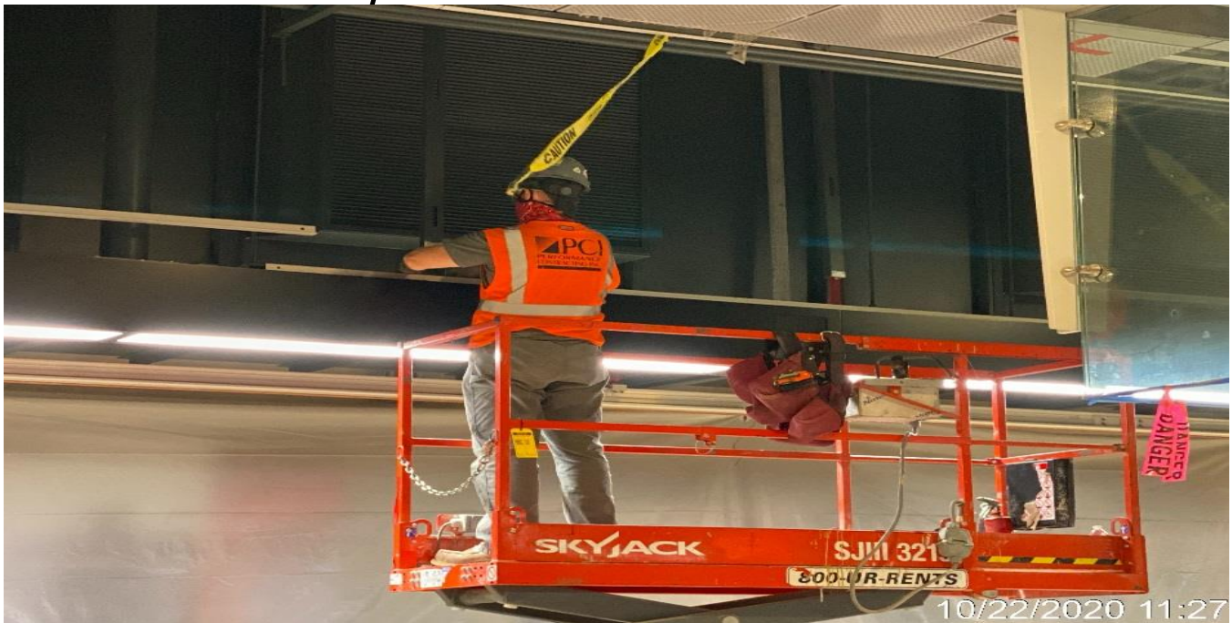
LEIMERT PARK STATION – Continue installing diagonal screen ceiling panels on the NB side of the platform.
