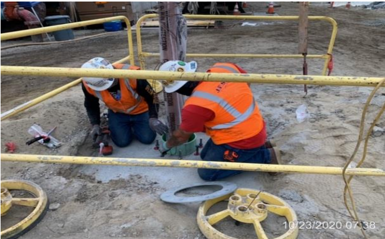
MLK STATION – Anchoring and aligning grating to Fresh Air Intake #1 at the plaza level.
