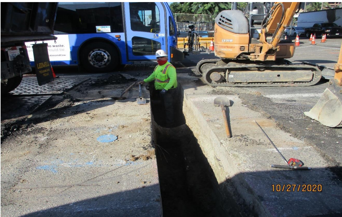
AVIATION/CENTURY- Trenching for traffic signal conduit on the south side of Aviation at Century.
