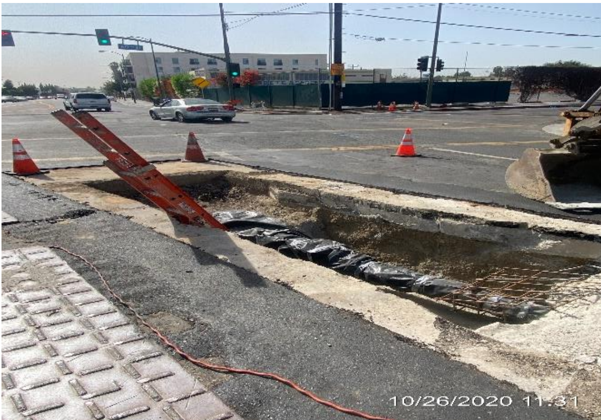
PARK MESA – Preparing to place concrete for the sub pump on southbound Crenshaw Blvd and 60th St.
