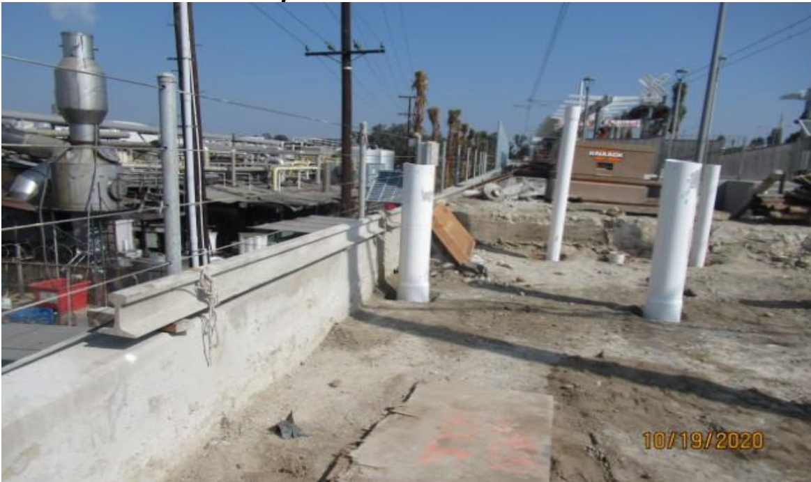
La Brea – La Brea wall 202 SB track WSCC has requested HCC to re-locate left rail into tie crib extending access deeper into platform area (looking north) Rework
