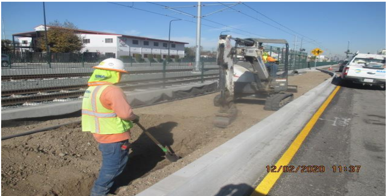
PARK MESA – Installing irrigation pipe line along the northbound median curb of Crenshaw Blvd starting on Slauson Ave and moving toward 57th St.
