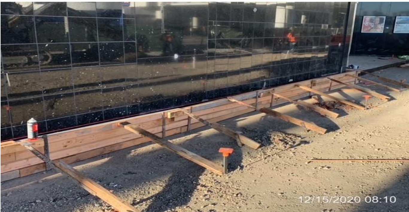
MLK STATION – Continue expansion board installation along the north side curb of the Mall at the plaza.
