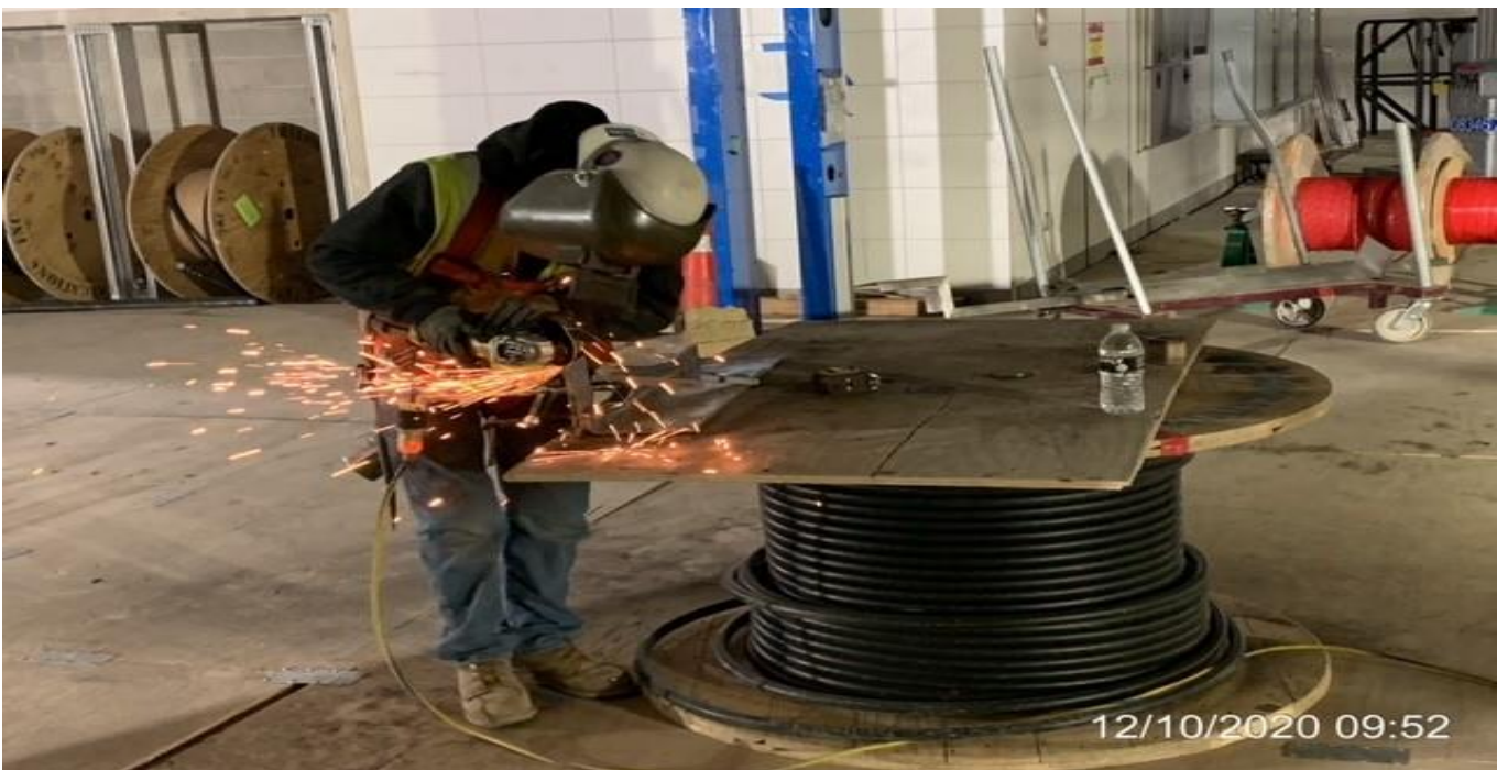
EXPO STATION – Fabricating for edge plate installation along the bottom guardrail perimeter of the escalator/staircase opening.
