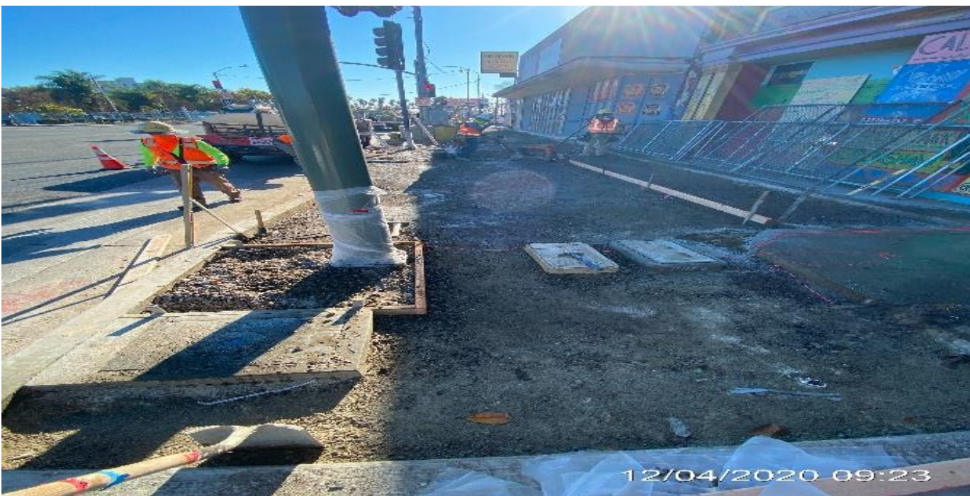
LEIMERT PARK STATION – Placing formwork for entire sidewalk on southbound Crenshaw Blvd between Vernon Ave and Homeland Dr.
