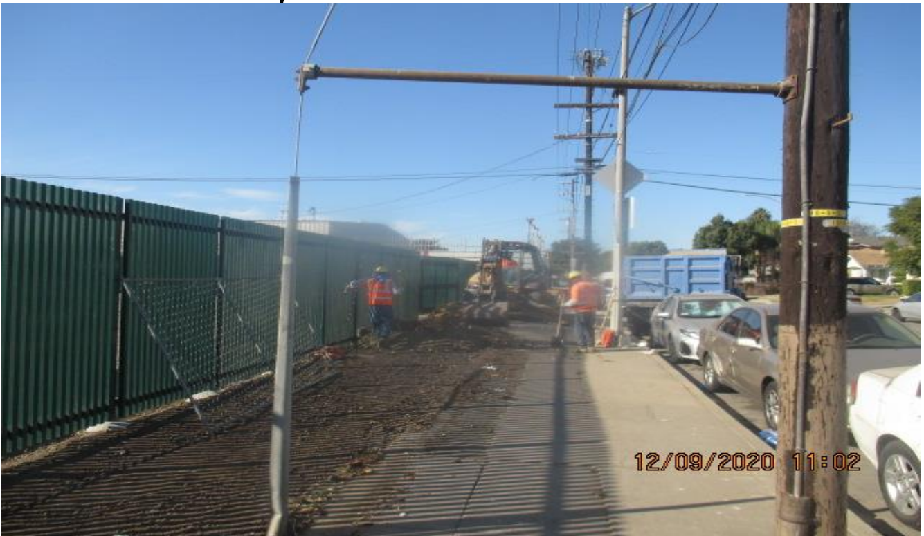
PARK MESA – Excavating/removing soil along the north portal fence of Victoria Auxiliary Site on eastbound 67th St in preparation for landscaping.
