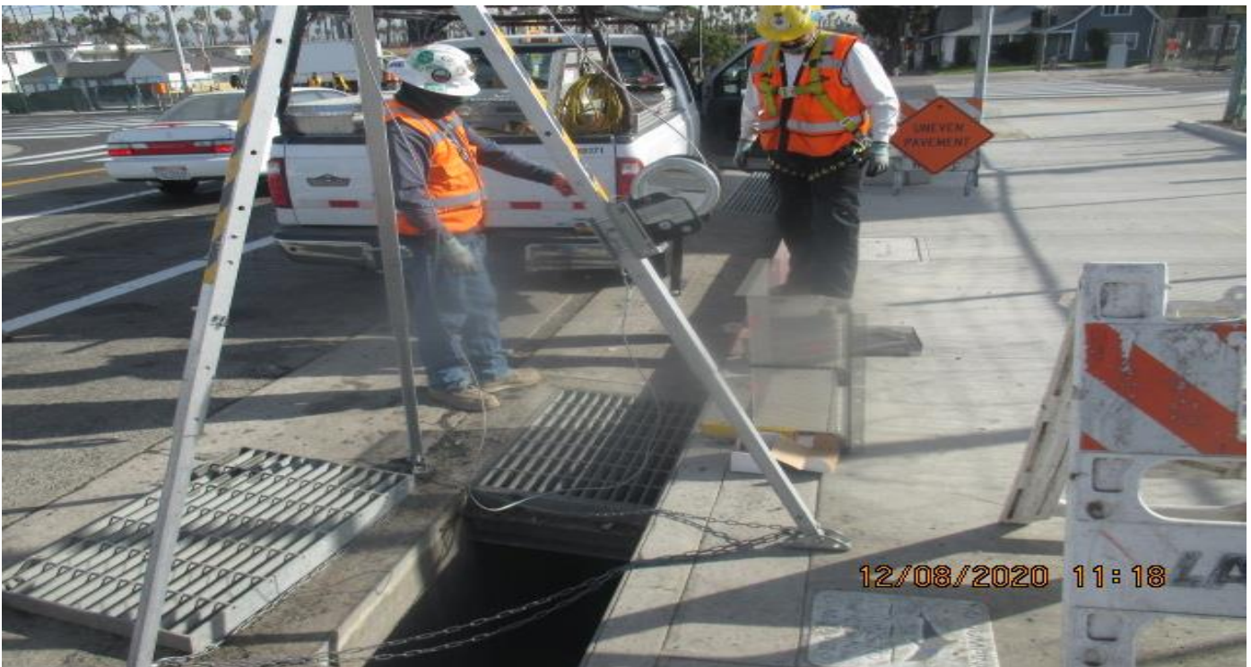
PARK MESA – Installing steel grates to Catch Basin #36 on the southwest corner of Crenshaw Blvd and 48th St.
