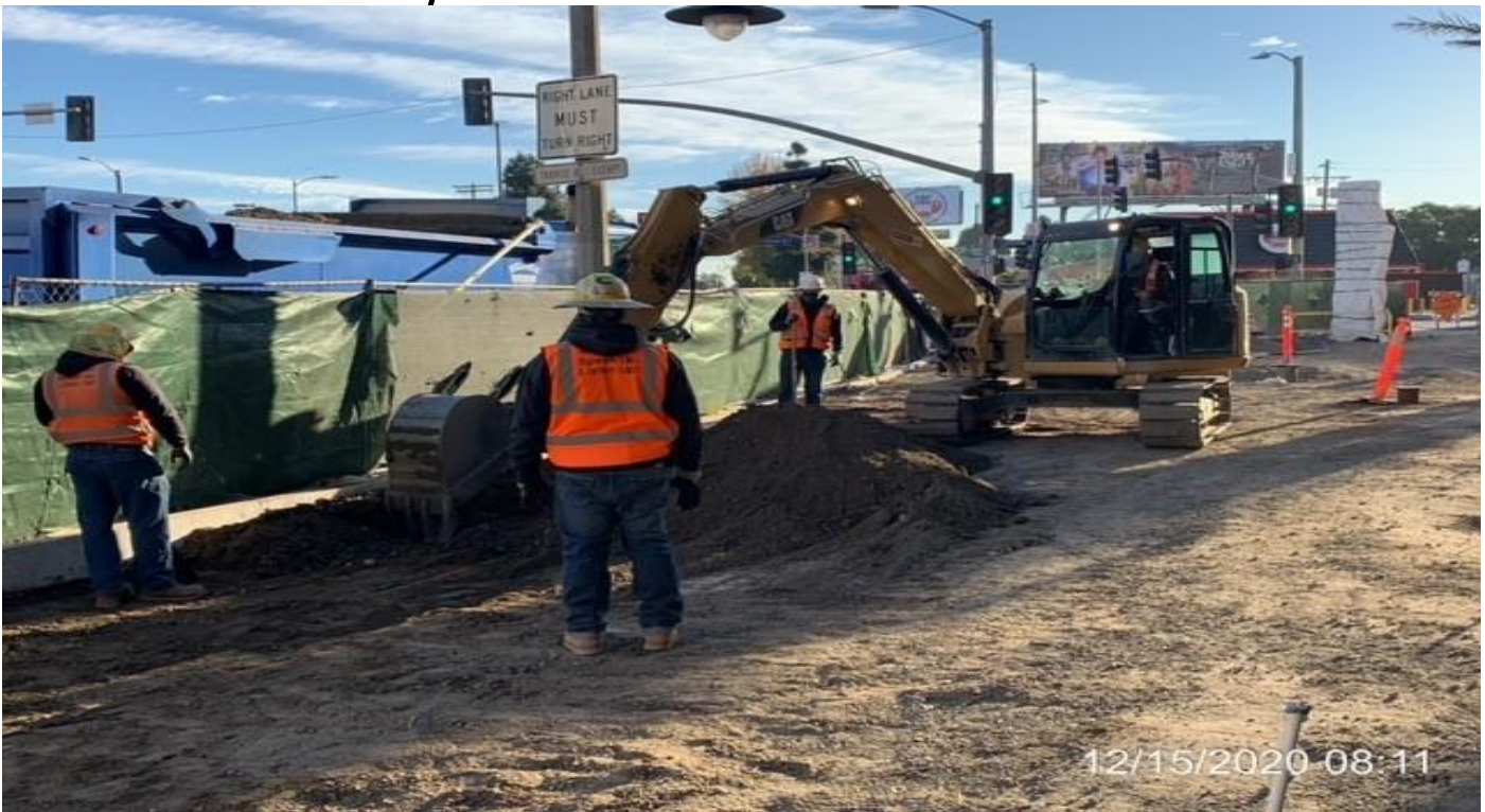
MLK STATION – Continue grading and compacting the far northwest area of the plaza.
