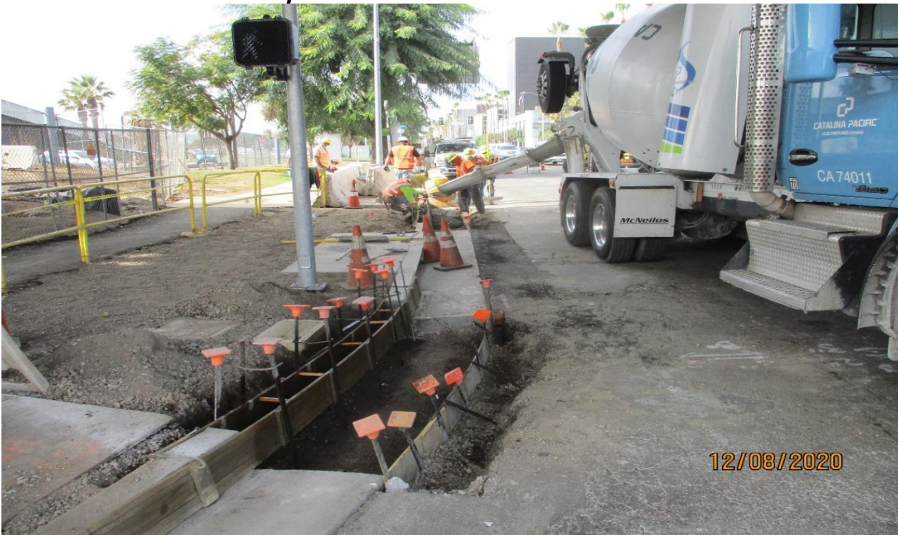
AVIATION/CENTURY- Placing curb and gutter concrete on the SW corner of Aviation and Century
