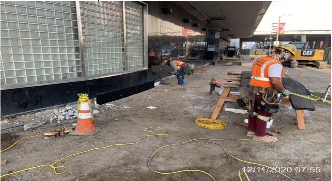
MLK STATION – Resume expansion board installation along the north side curb of the Mall at the plaza.
