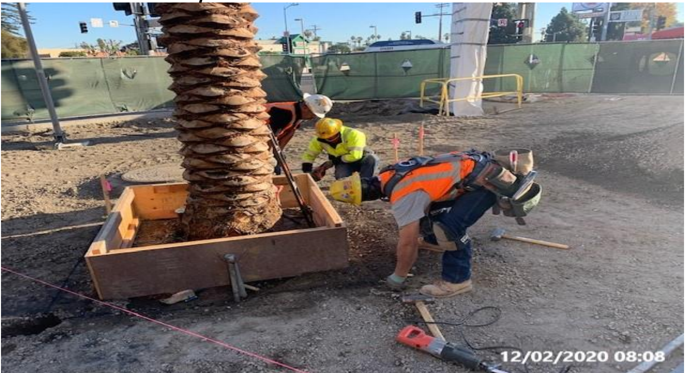
MLK STATION – Building formwork for steel grate frame installation around palm tree bases at the plaza.
