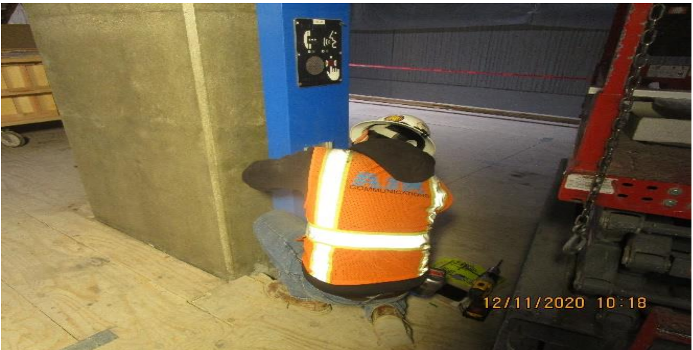
MLK STATION – Drilled and anchored passenger telephone pedestal at the north end of the platform.
