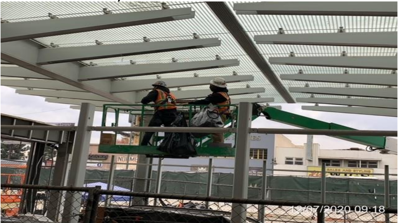
MLK STATION – Continue caulking and sealing the BOCA light fixtures at the main entrance canopy of the plaza.
