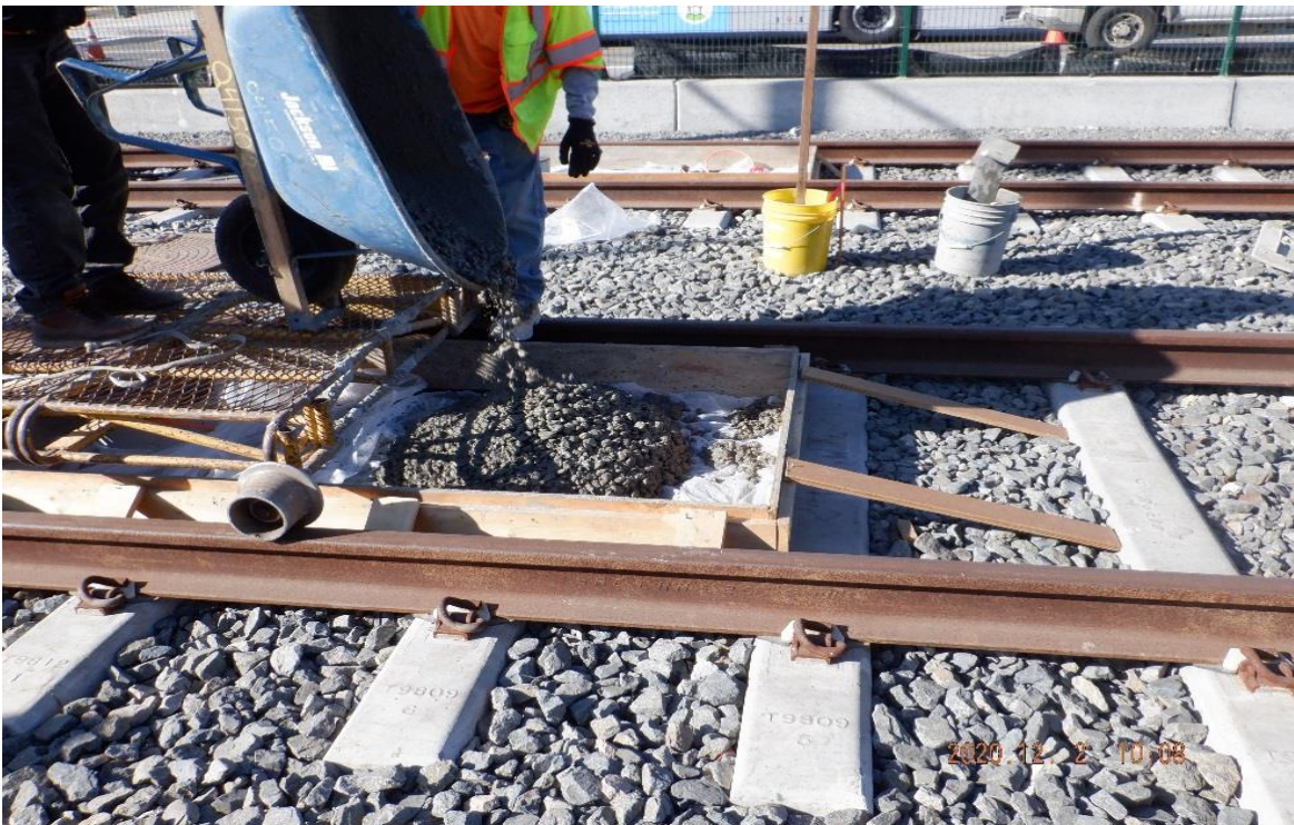
PARK MESA – STA 339+70 TK#4/NB looking west – traffic loop detector slab PCC pour – north of 54th St at grade Xing.
