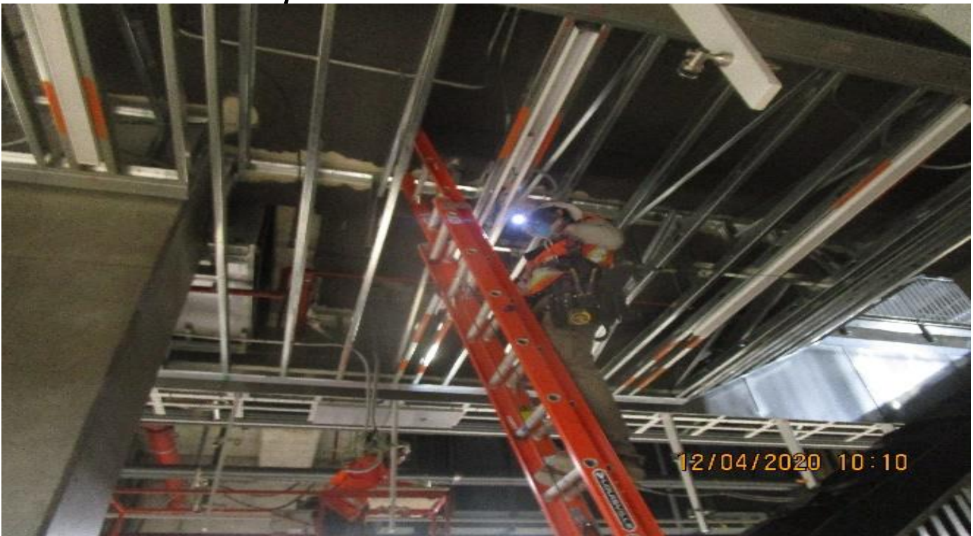
MLK STATION – Installing LED light fixtures above Escalator 3 and Staircase 2 at the platform.
