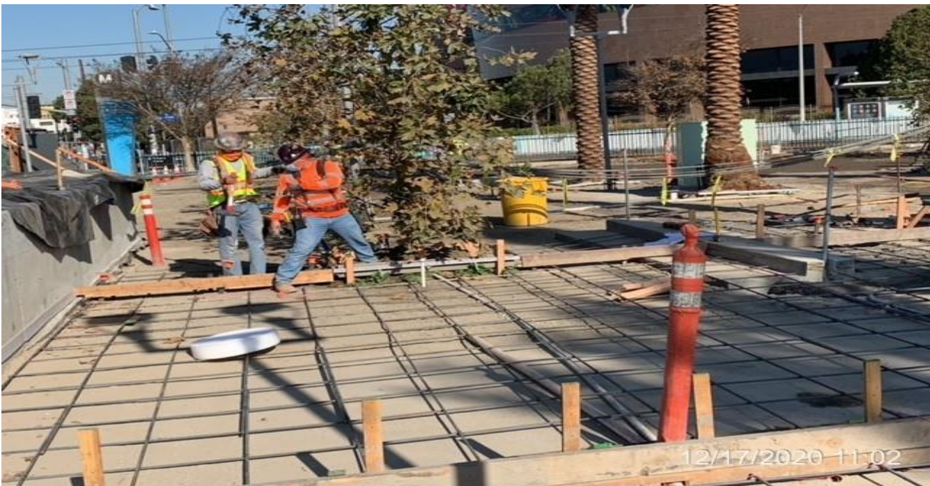
EXPO STATION – Continue building formwork and placing rebar for the architectural topping slab at the north end of the station.
