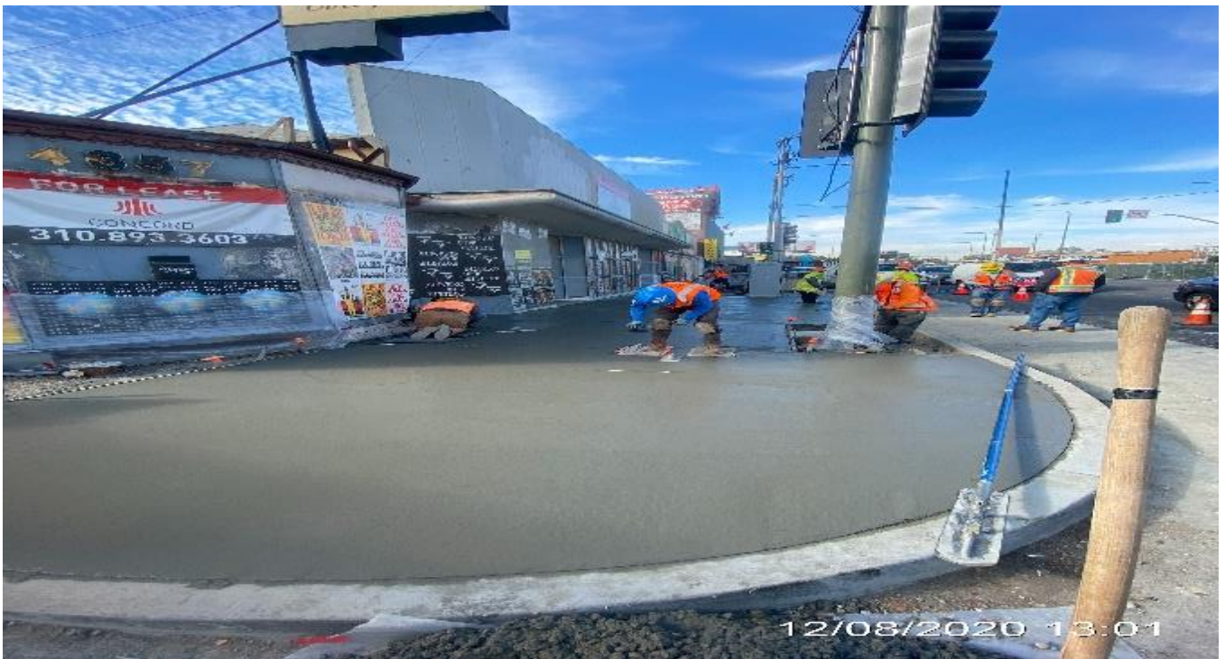
LEIMERT PARK STATION – Placing concrete for the entire sidewalk on southbound Crenshaw Blvd between 43rd Pl and Homeland Dr.
