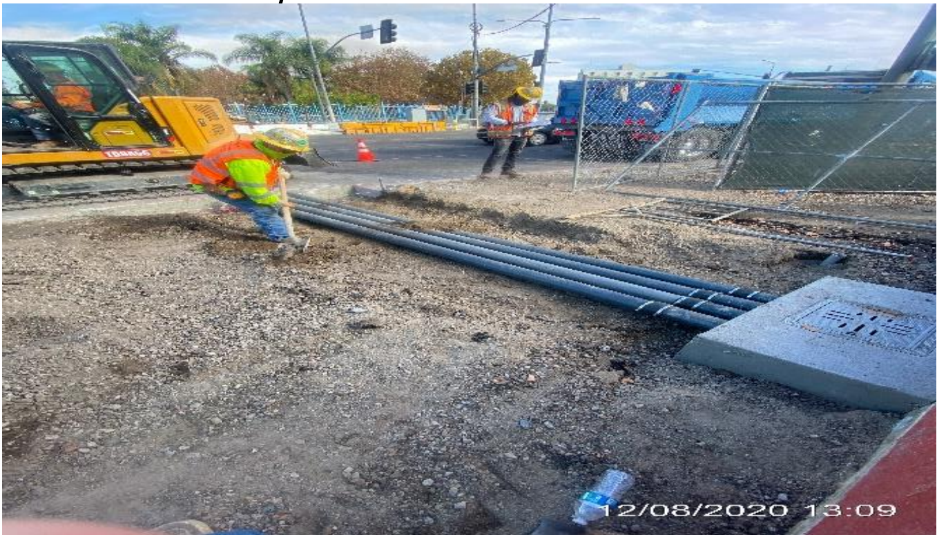
LEIMERT PARK STATION – Installing PVC pipes to the culvert drainage on the northwest corner of Crenshaw Blvd and Vernon Ave.
