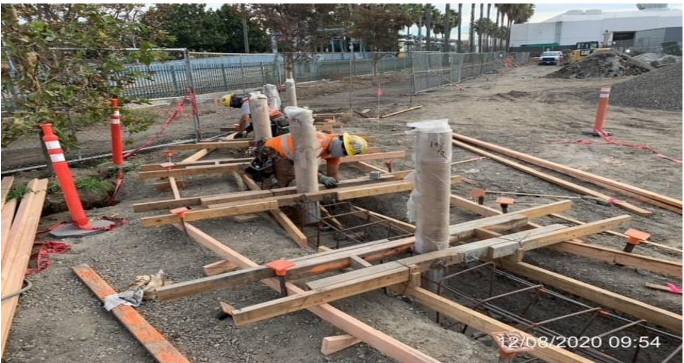
EXPO STATION – Continue setting formwork and installing the remaining steel bollards at the north end of the plaza.
