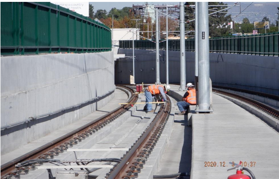
UG4 – STA 365+20 TK#3/SB looking north – shimming curve SB-33 of UG4 south portal.
