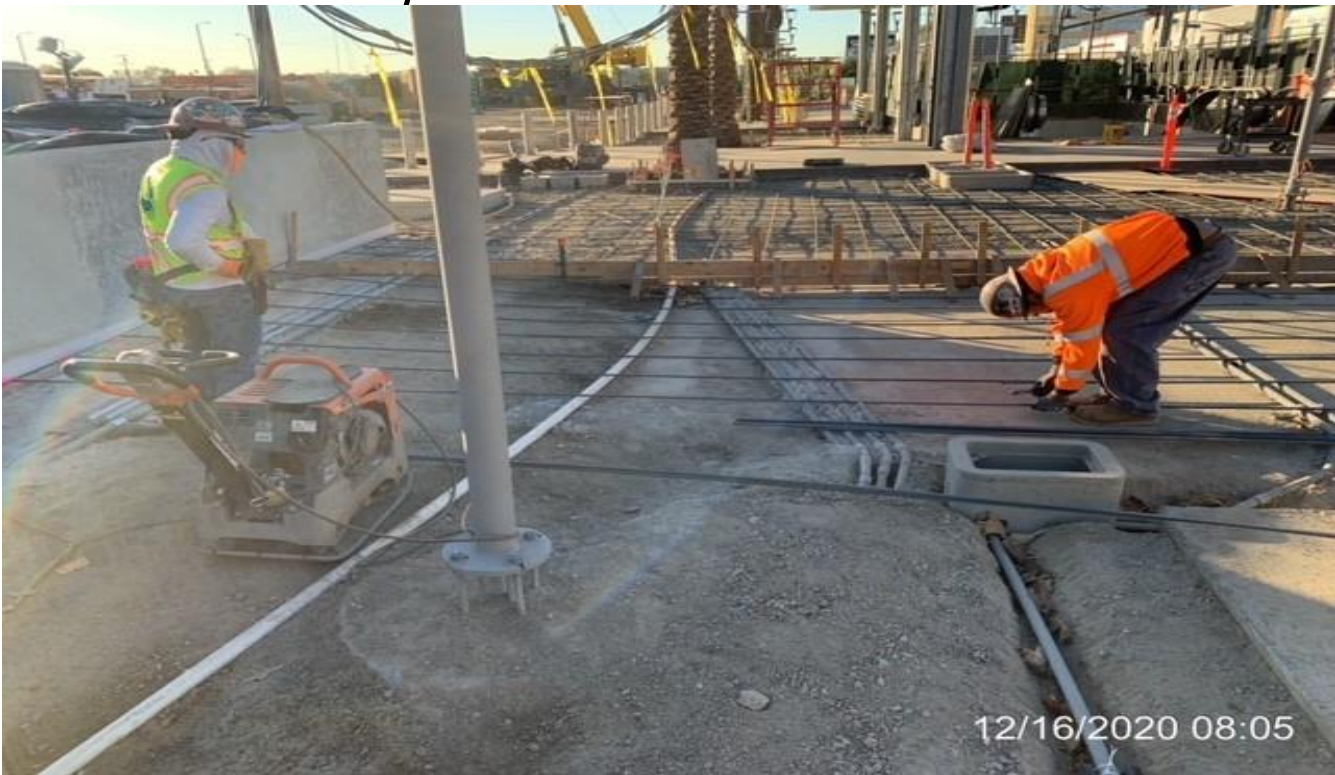
EXPO STATION – Resume building formwork and placing rebar for the architectural topping slab at the north end of the station.
