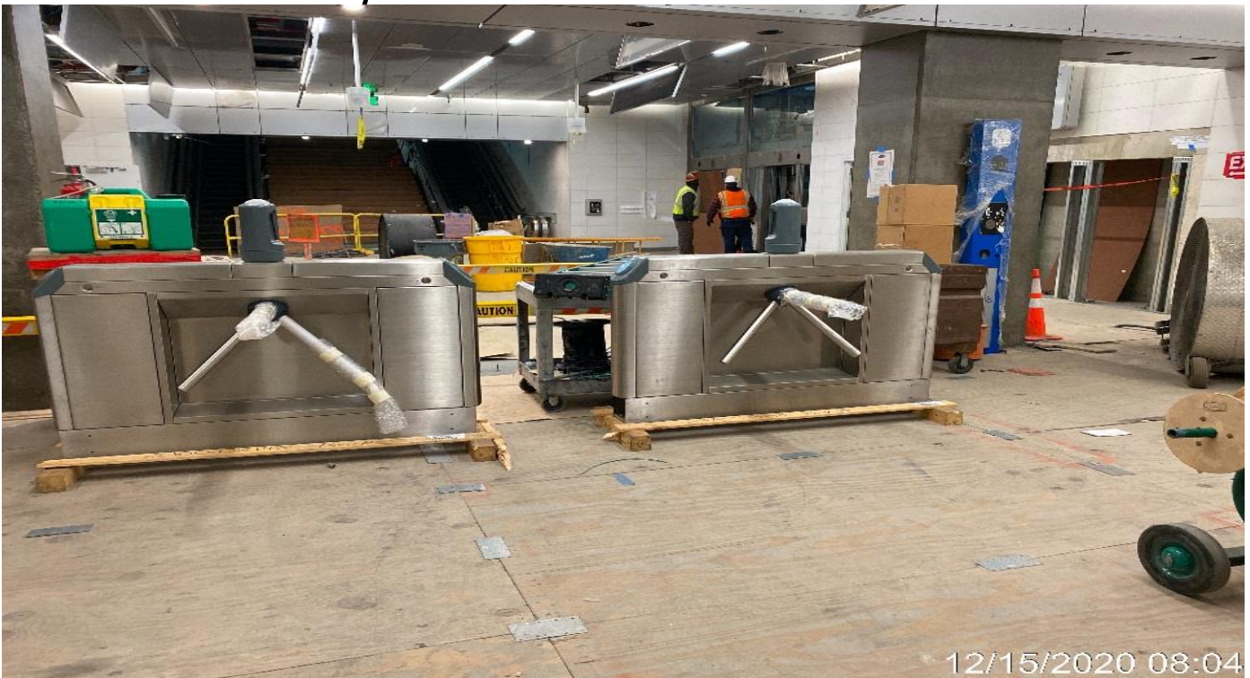
LEIMERT PARK STATION – Installing fare gate turnstiles at the concourse Paid Area C-146.
