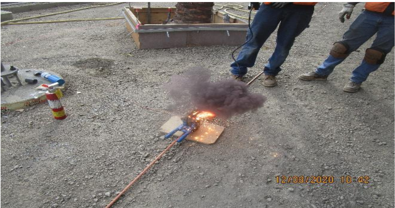
MLK STATION – Continue installing ground grid system at the north end section of the plaza.
