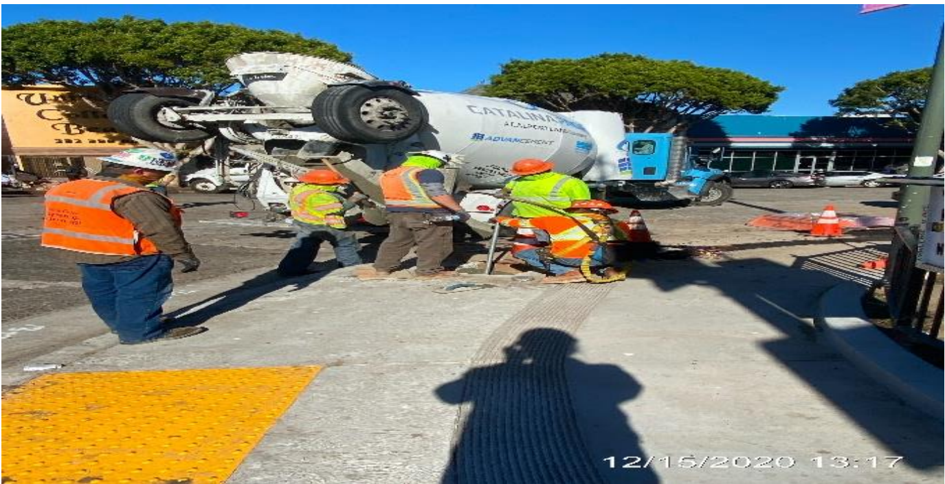
LEIMERT PARK STATION – Placing concrete for street light foundation on the southeast corner of Crenshaw Blvd and 43rd Pl.
