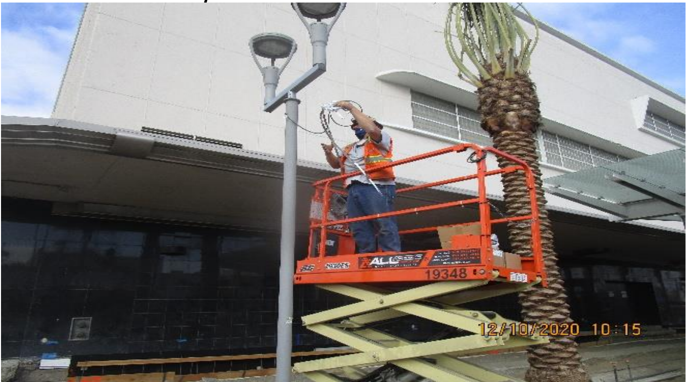
MLK STATION – Installing CCTV support brackets to the pedestrian light poles at the plaza.
