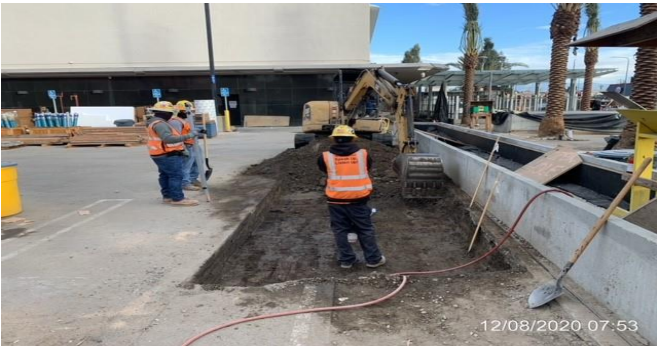
MLK STATION – Continue excavating for curb and gutter trench drain along the south service road of the plaza.
