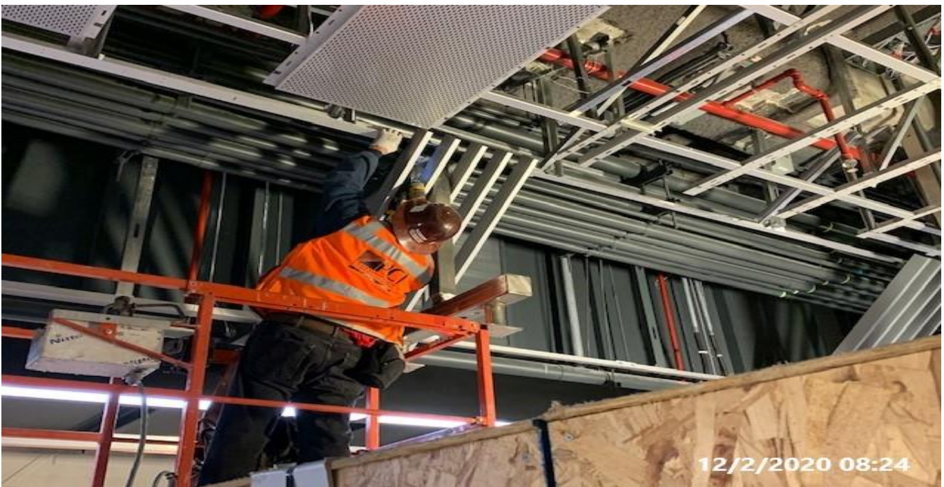
MLK STATION – Installing diagonal screen ceiling panels along the northbound side of the platform.
