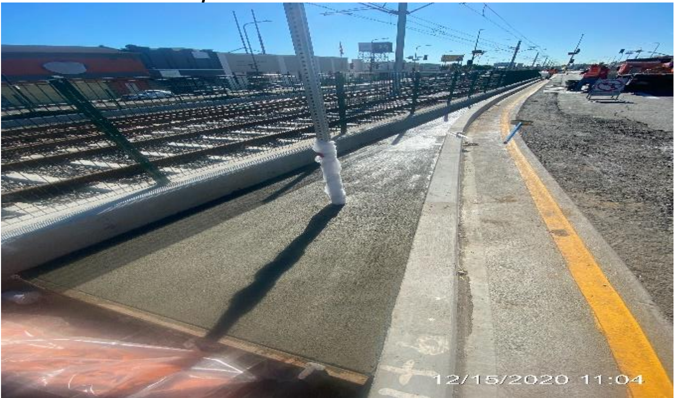
PARK MESA – Placing cobble mortar base to the southbound median curb of Crenshaw Blvd from 57th St to 54th St.
