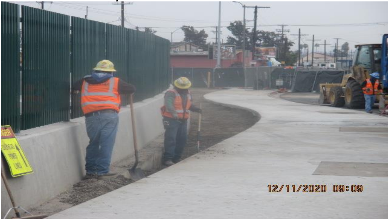
PARK MESA – Excavating/removing soil on eastbound New Road along the northbound barrier wall of UG3 in preparation for landscaping.
