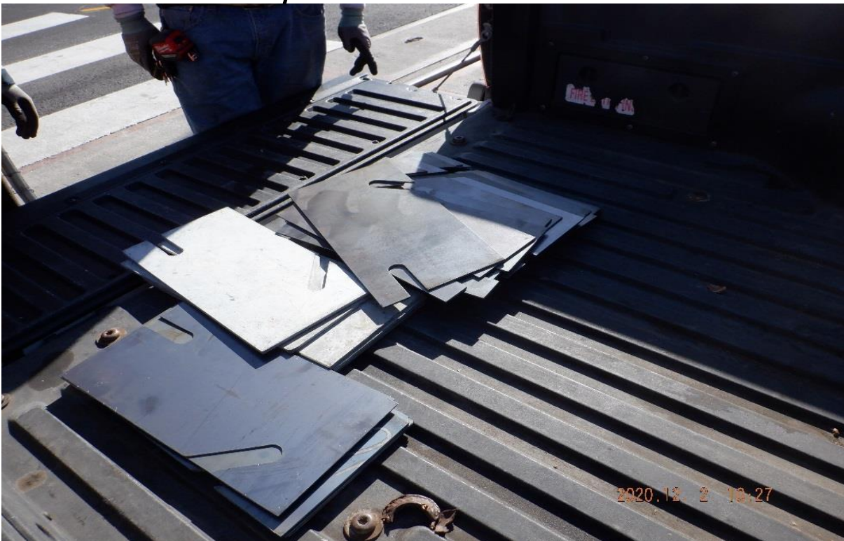
UG4 – STA 364+00 TK#4/NB – shim material delivered in UG4 does not look to be galvanized steel nor stainless steel (left & right pile)
