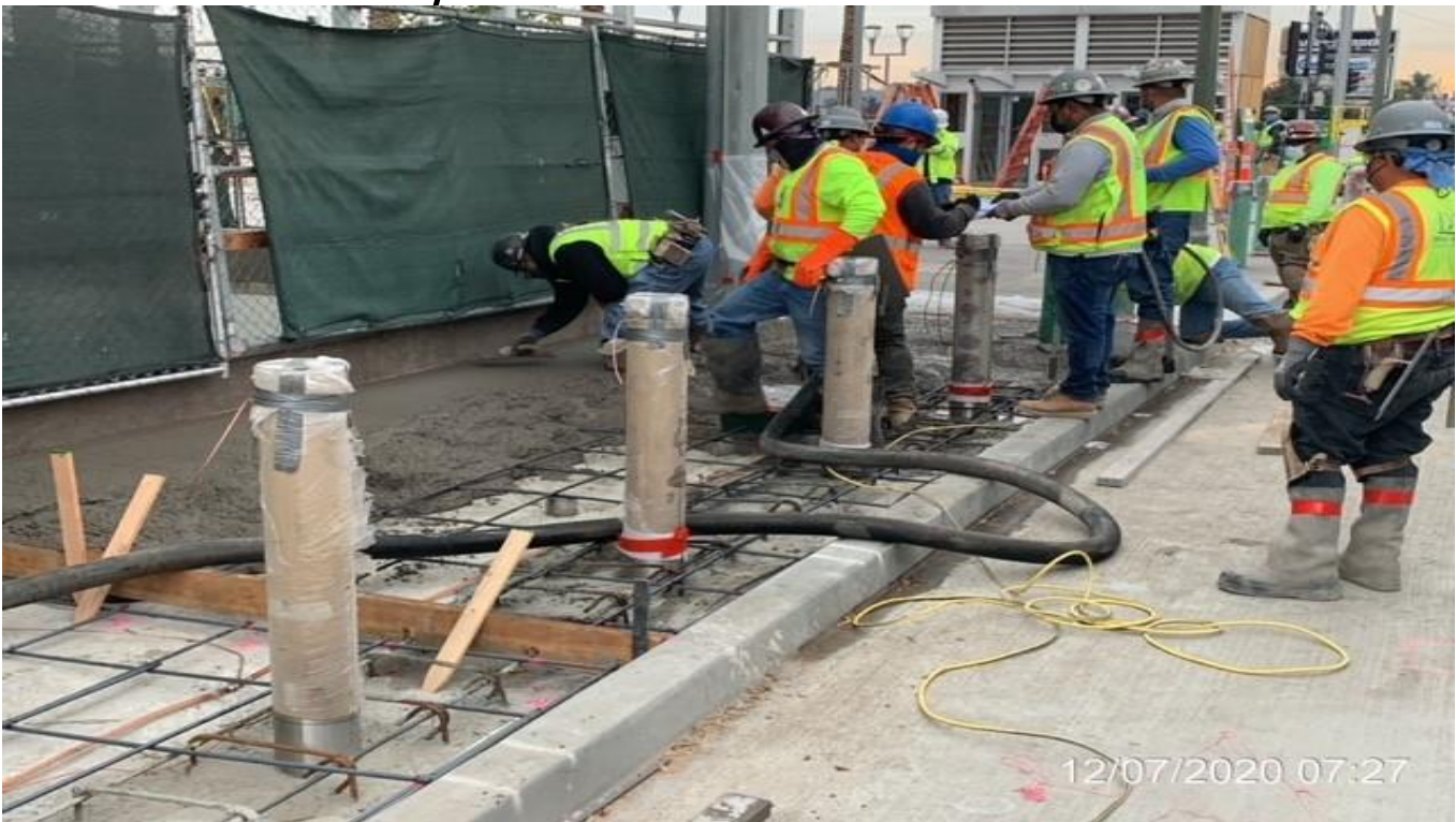
EXPO STATION – Placing concrete for the architectural topping slab at the north end of the plaza.
