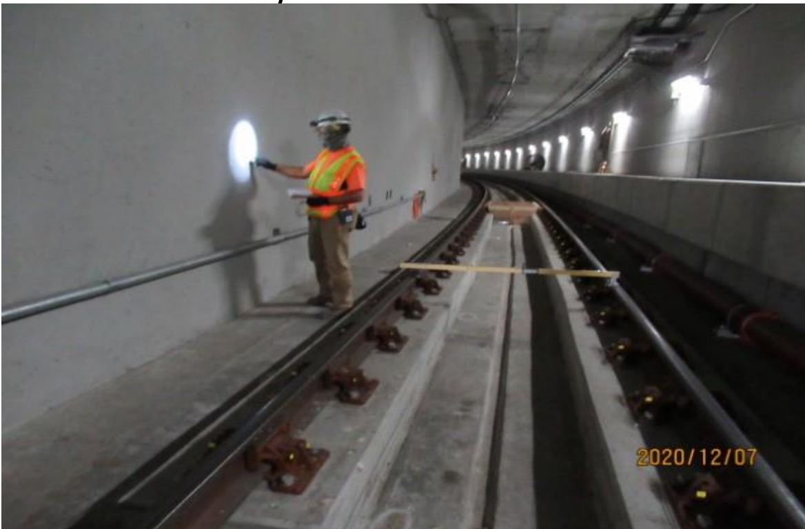
UG4 – Metro's QA Track Inspector on SB track in UG4 verifying correct survey spiral locations for SB-34 curve (looking north)
