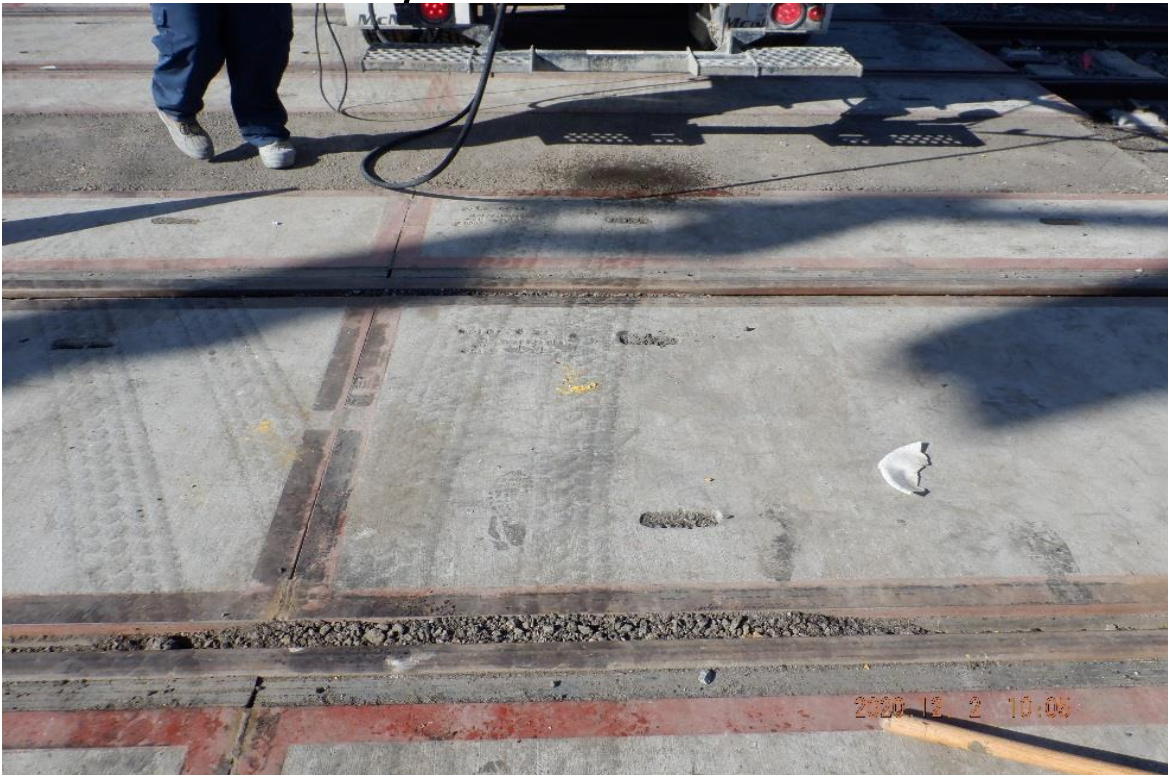
PARK MESA – STA 339+19 TK#4/NB looking west – AC in the crossing panel flangeway after road improvement work on Crenshaw Blvd with 54th St
