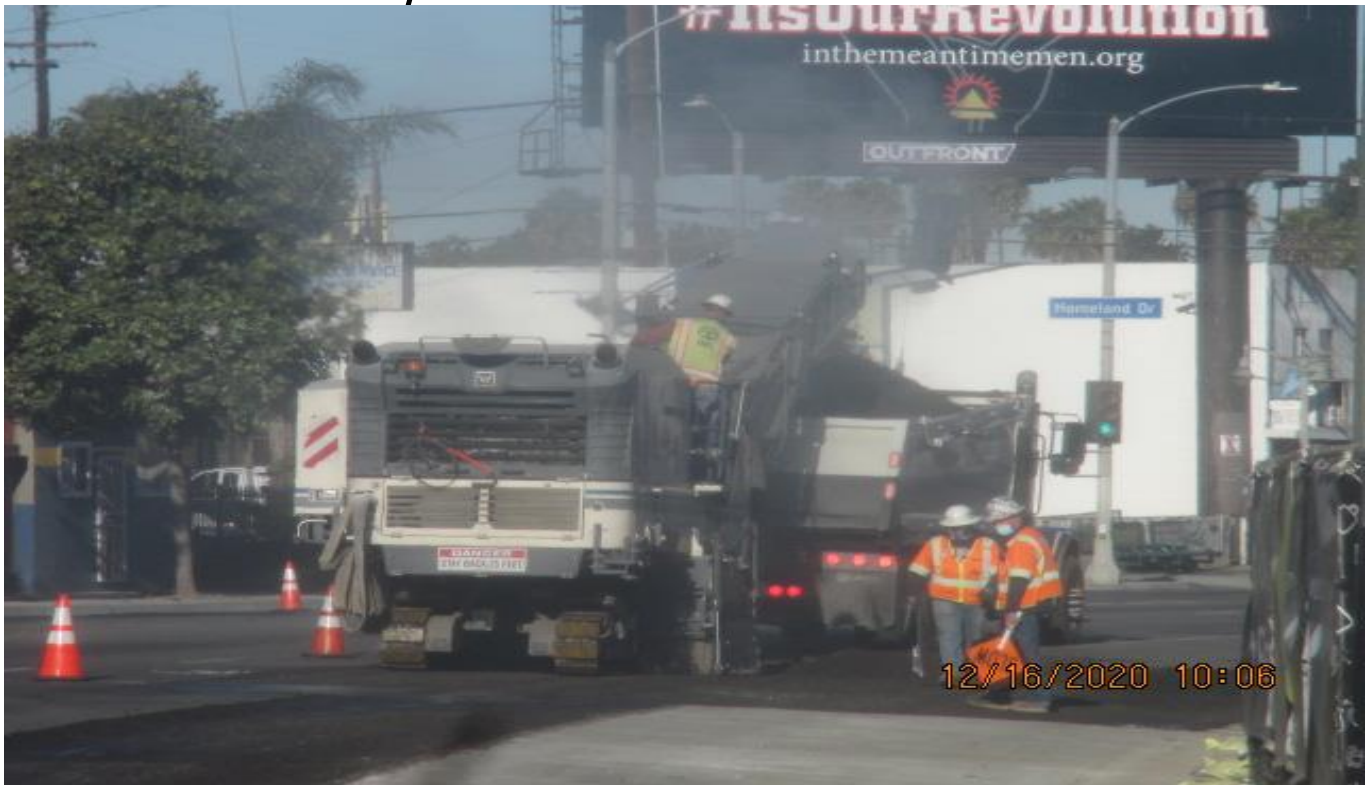
LEIMERT PARK STATION – Placing asphalt concrete along northbound Crenshaw Blvd starting from Vernon Ave and ending at Homeland Dr
