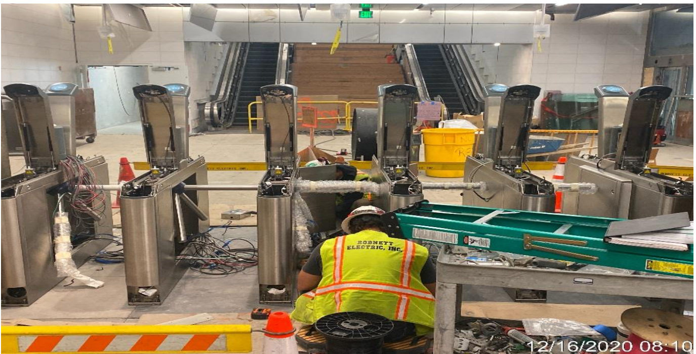
LEIMERT PARK STATION – Continue installing fare gate turnstiles at the concourse Paid Area C-146.
