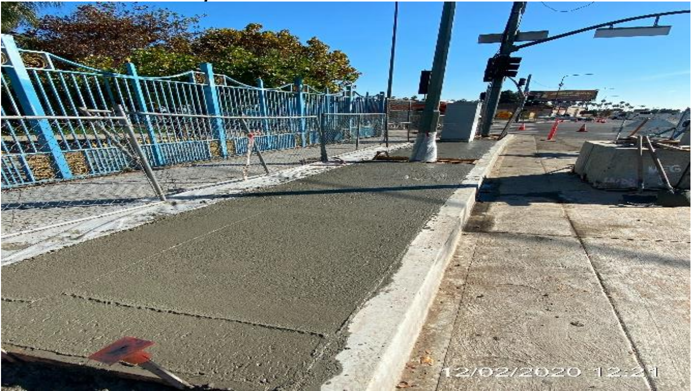
LEIMERT PARK STATION – Placed concrete over sidewalk on northbound Crenshaw Blvd between Vernon Ave and 43rd Pl.
