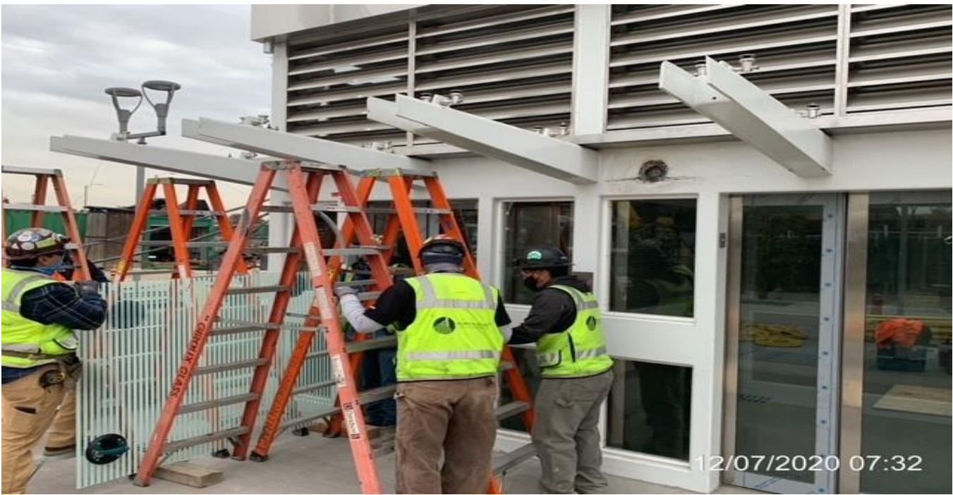
EXPO STATION – Installing glass panels to the top section of Elevators 1&2 at the plaza.
