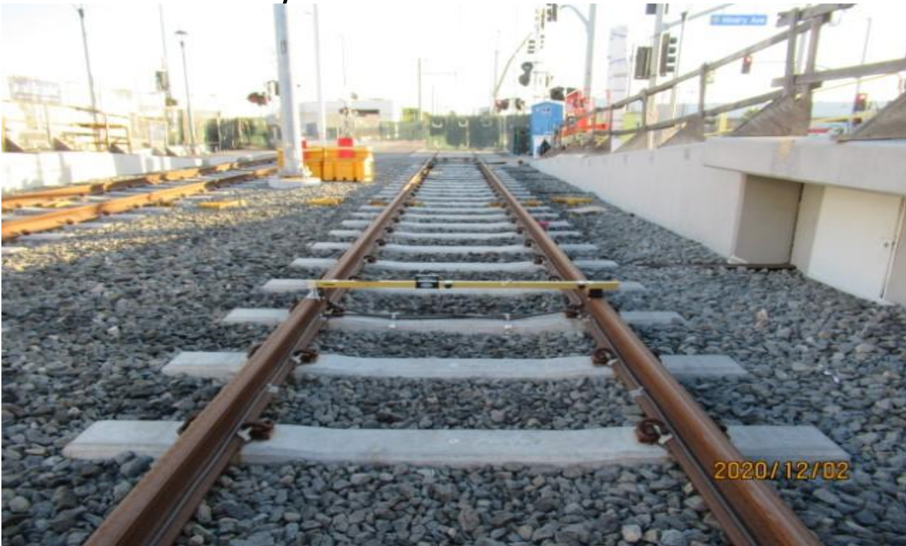
Hindry – Verifying cross levels at Hindry Station NB track STA 134+59 (looking north) Re-tamped by HCC
