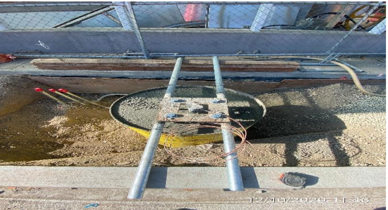
MLK STATION – Placed concrete for street light foundations along the east side of the plaza.
