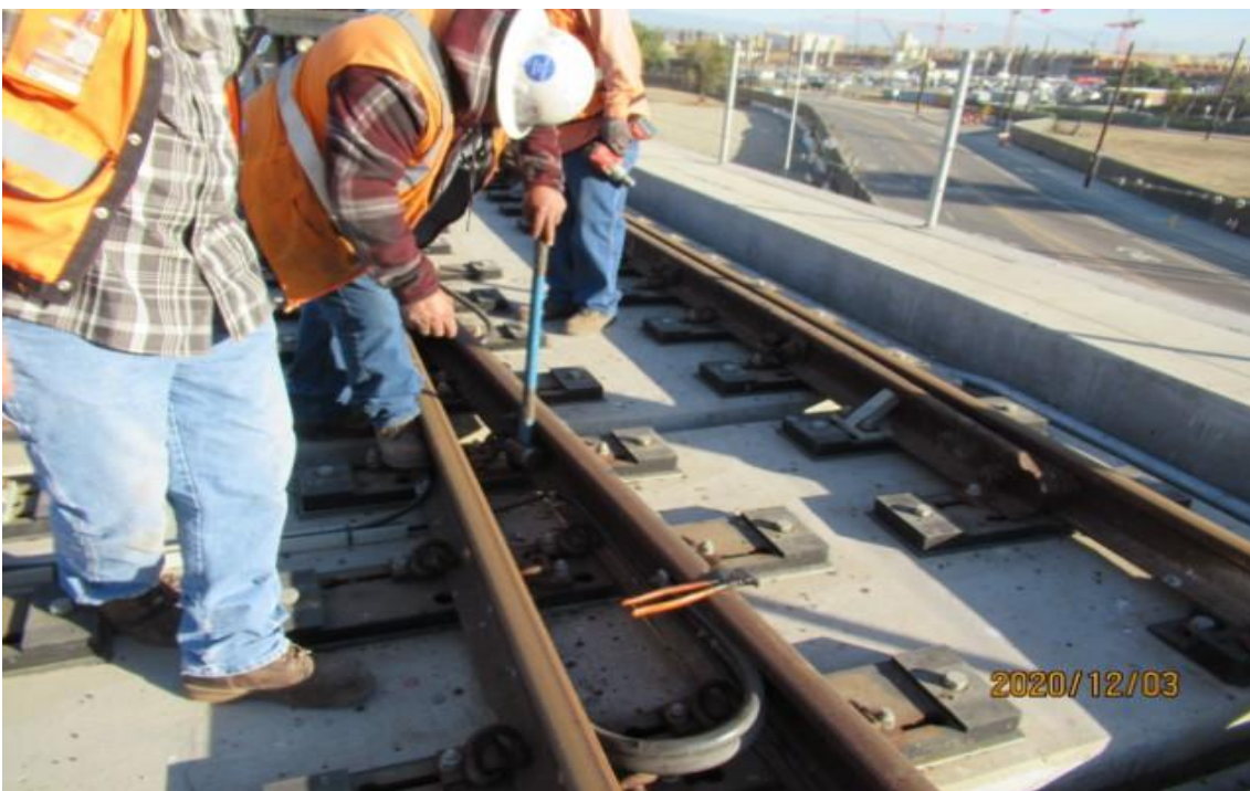
AVIATION/CENTURY- HCC working on 10K1LHXO open issues log for NB track Century/Aviation bridge (looking northeast) Rework
