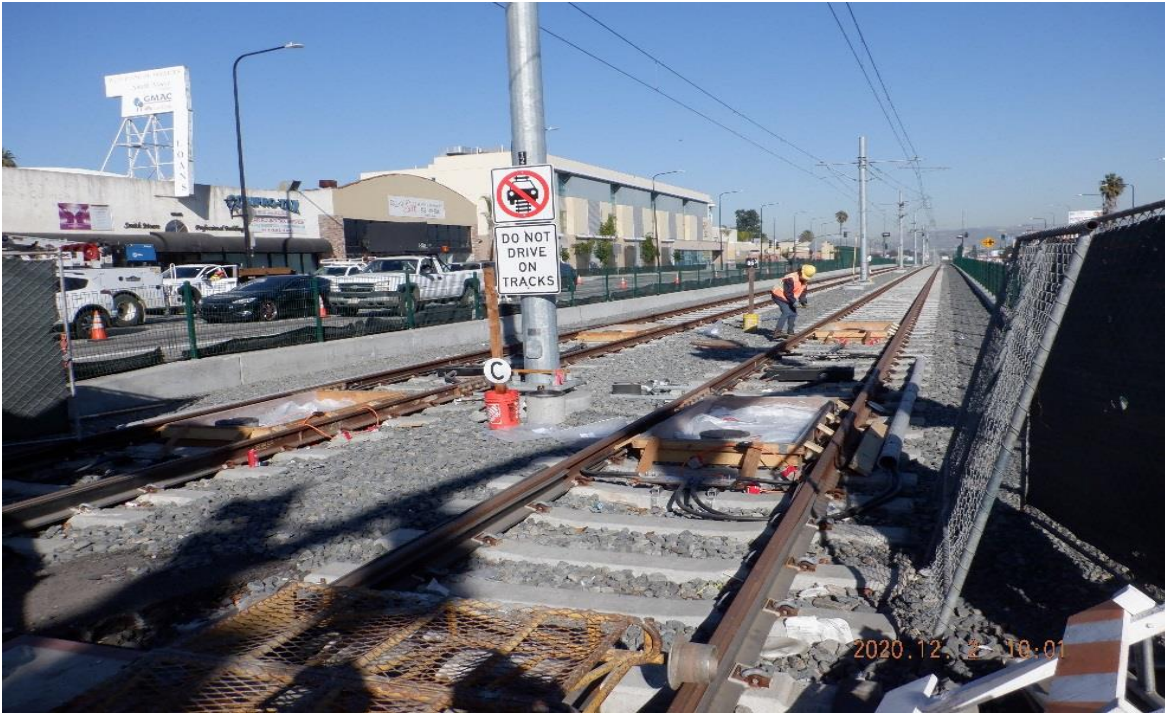
PARK MESA – STA 339+40 TK#4,NB looking north – site north of 54th St at grade Xing – traffic loop detector slab forms between rails ready to receive PCC
