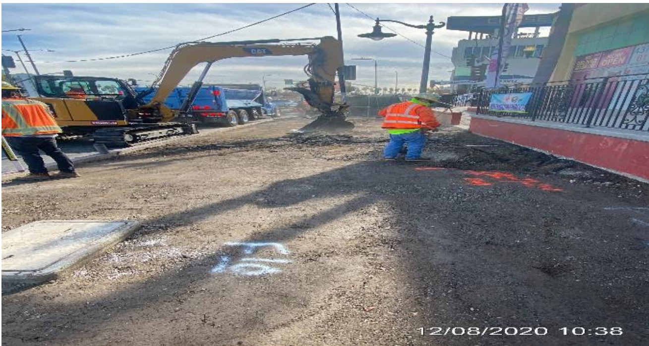
LEIMERT PARK STATION – Continue backfilling and compacting the entire sidewalk on southbound Crenshaw Blvd between Vernon Ave and Homeland Dr.
