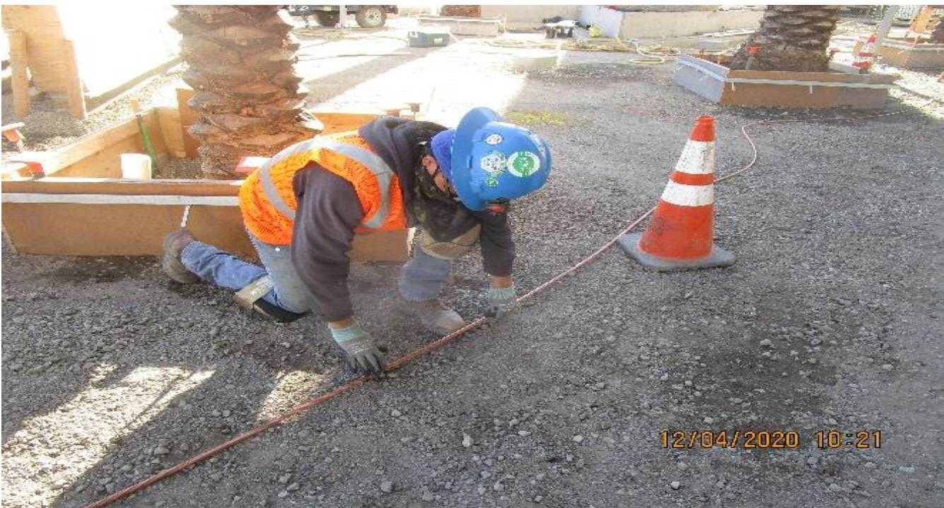
MLK STATION – Installing ground grid system at the north end section of the plaza.
