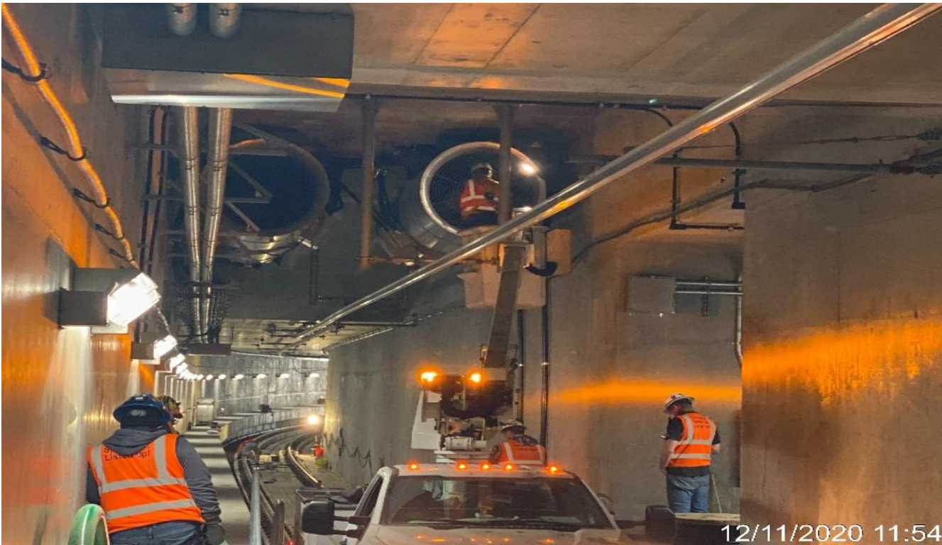
UG3 – Performing pre-start up inspections to the tunnel booster fans on the southbound tunnel.
