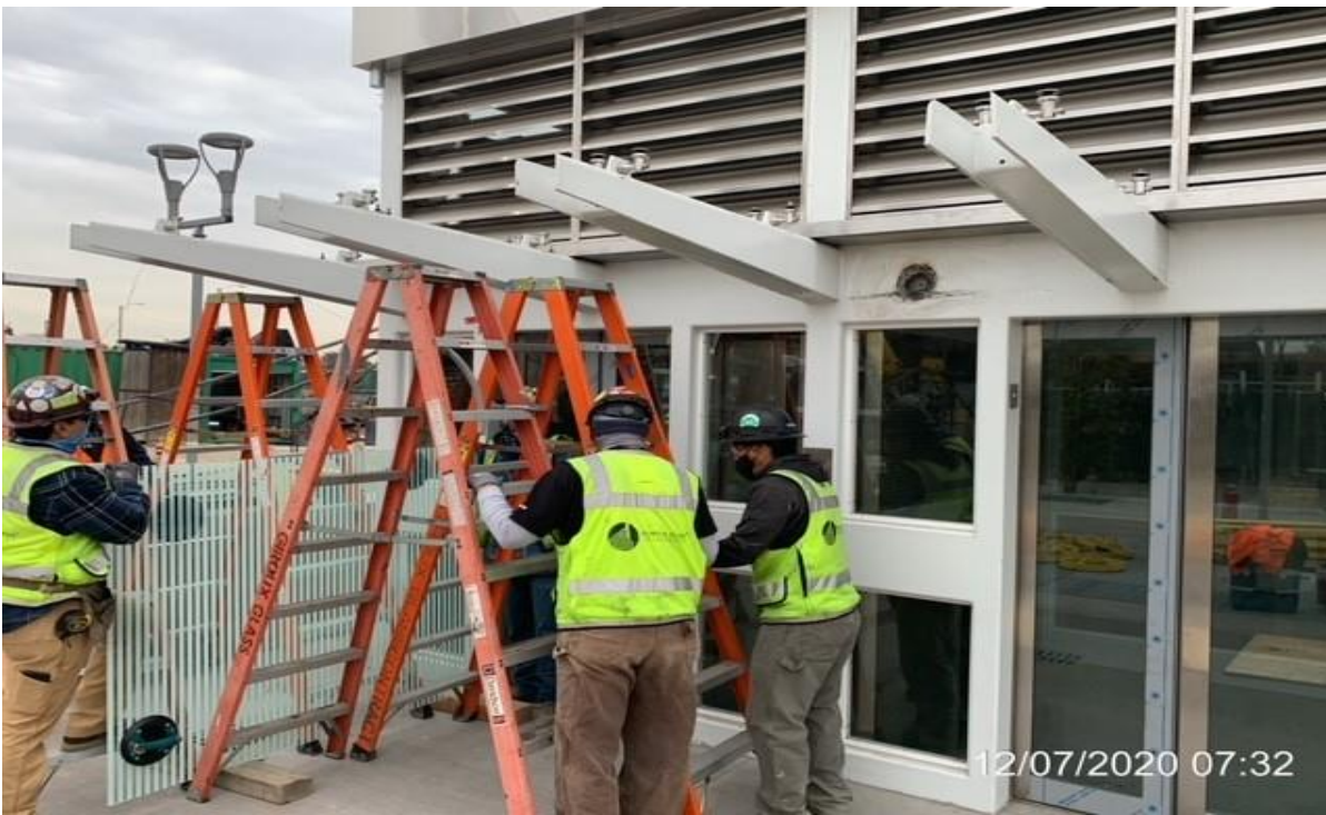
EXPO STATION – Giroux Glass installing glass for eyebrow on elevator structure #1 and #2
