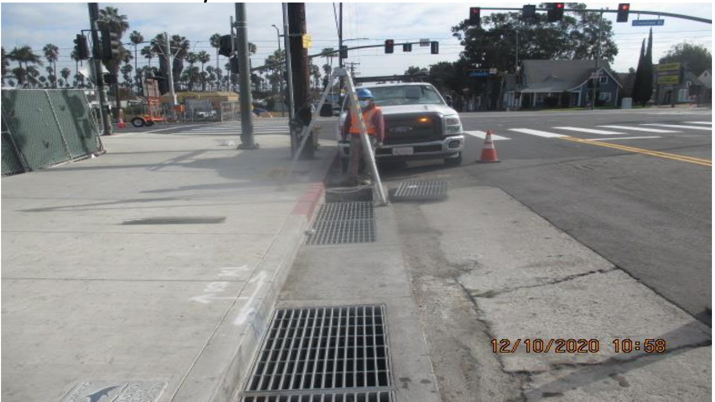
PARK MESA – Installing steel grates to Catch Basin #29 and #37 on eastbound 48th St and Crenshaw Blvd.
