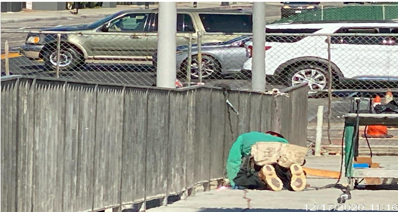
PARK MESA – Continue installing guardrails along the north and southbound side of the north end entrance ramp.
