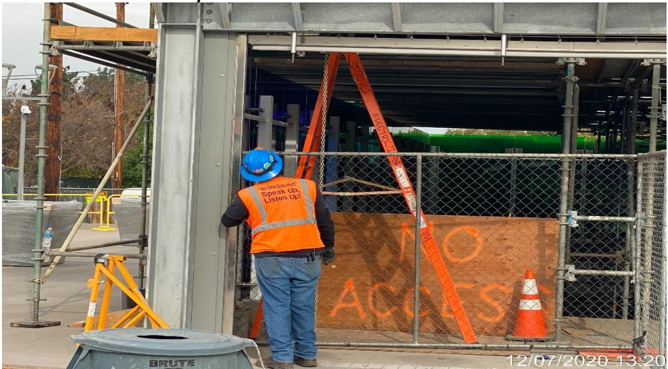
LEIMERT PARK STATION – Performing electrical work to the main entrance roll-up gate at the plaza.
