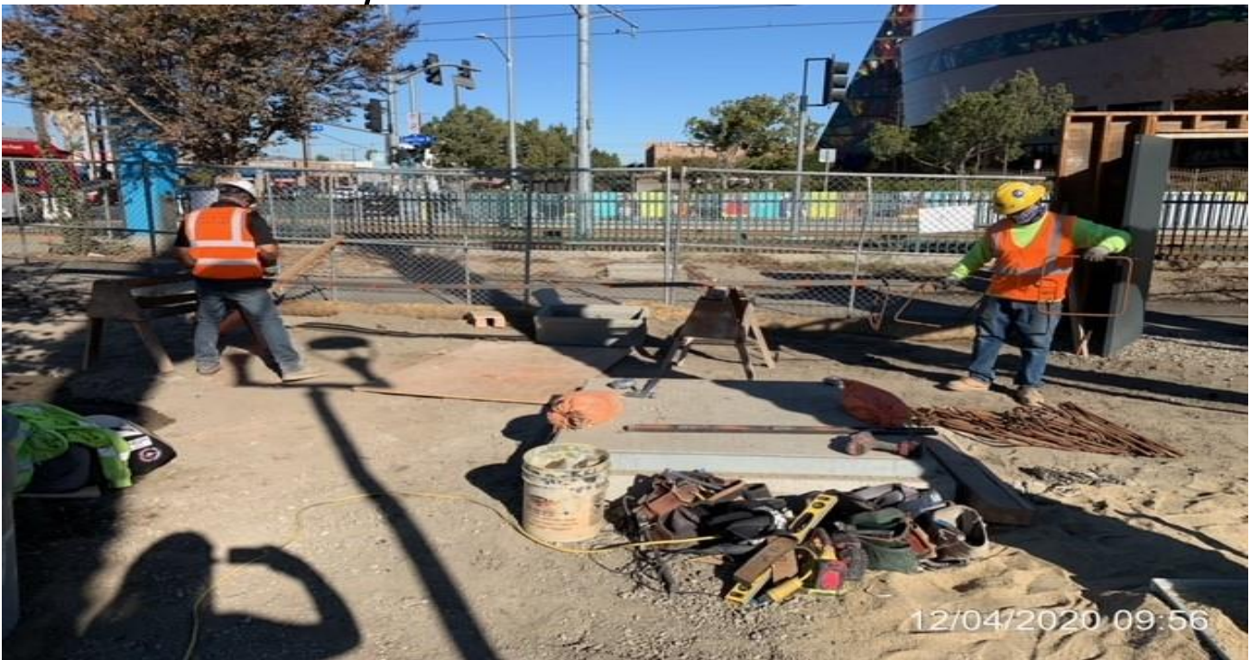
EXPO STATION SITE– Building formwork for the remaining steel bollard foundations at the north end of the plaza.
