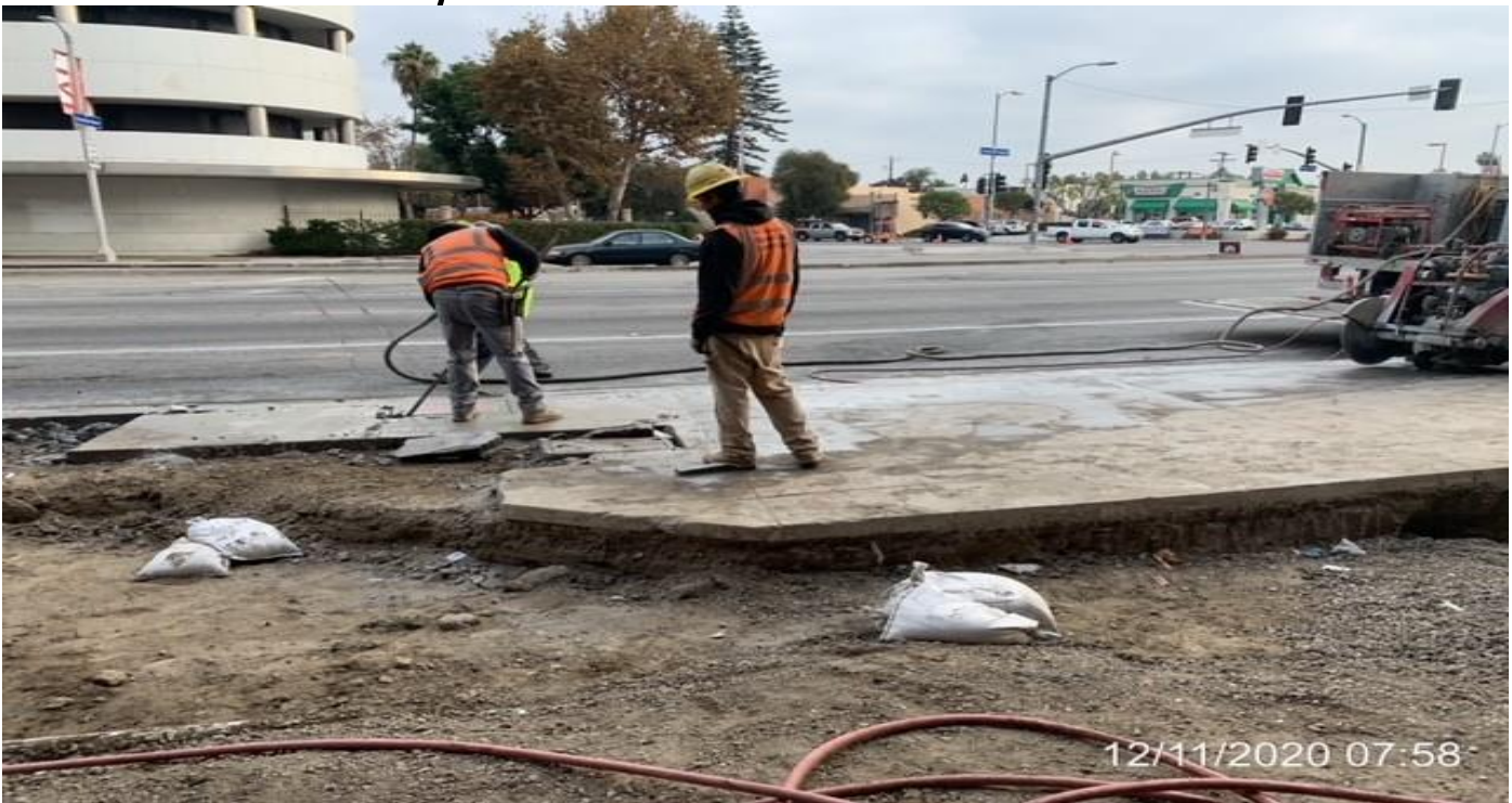
MLK STATION – Continue demolishing and removing remaining sidewalk sections at the far northwest area of the plaza.
