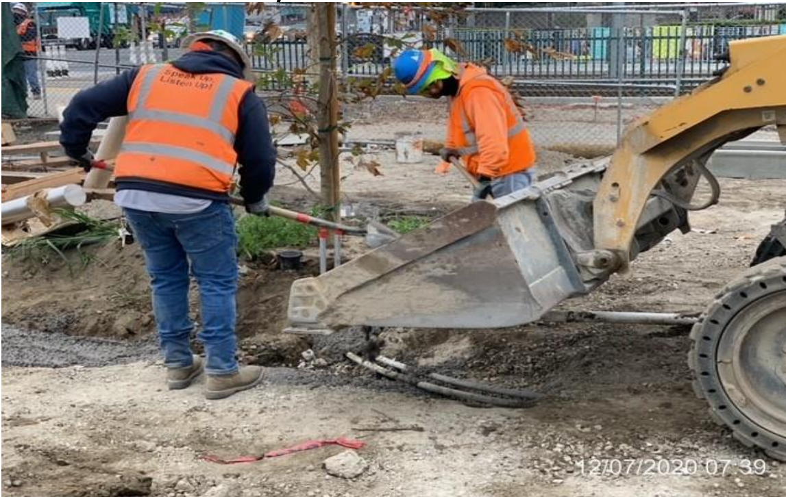
EXPO STATION – WSCC crew concrete encasing electrical conduit for palm tree lighting.
