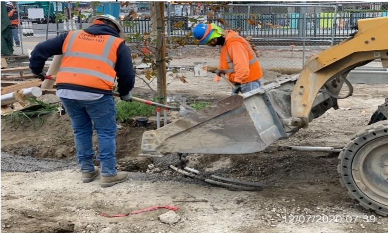
EXPO STATION – Concrete encasing landscape lighting conduit for trees at the plaza.
