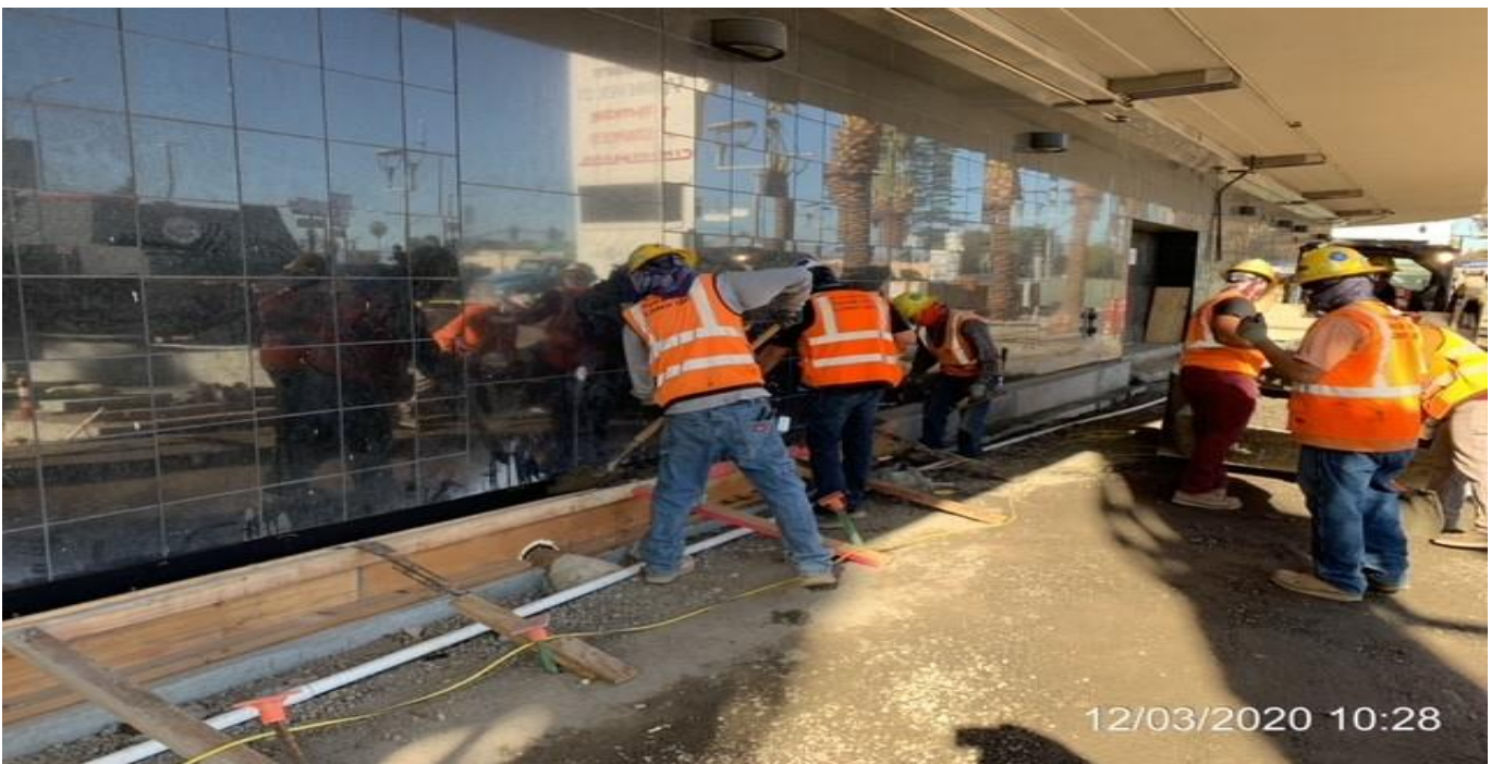
MLK STATION – Placing concrete for the walkway curb along the entire east side of the Mall at the plaza.
