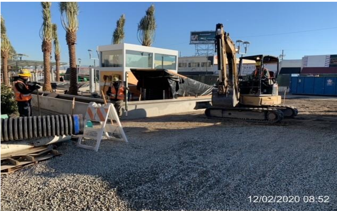
MLK STATION – Excavating for curb and gutter trench drain along the south service road of the plaza.
