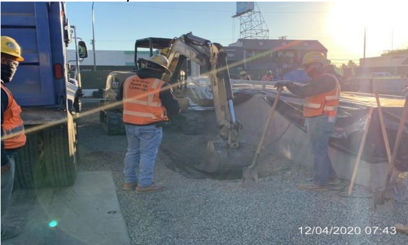
MLK STATION – Continue excavating for curb and gutter trench drain along the south service road of the plaza.
