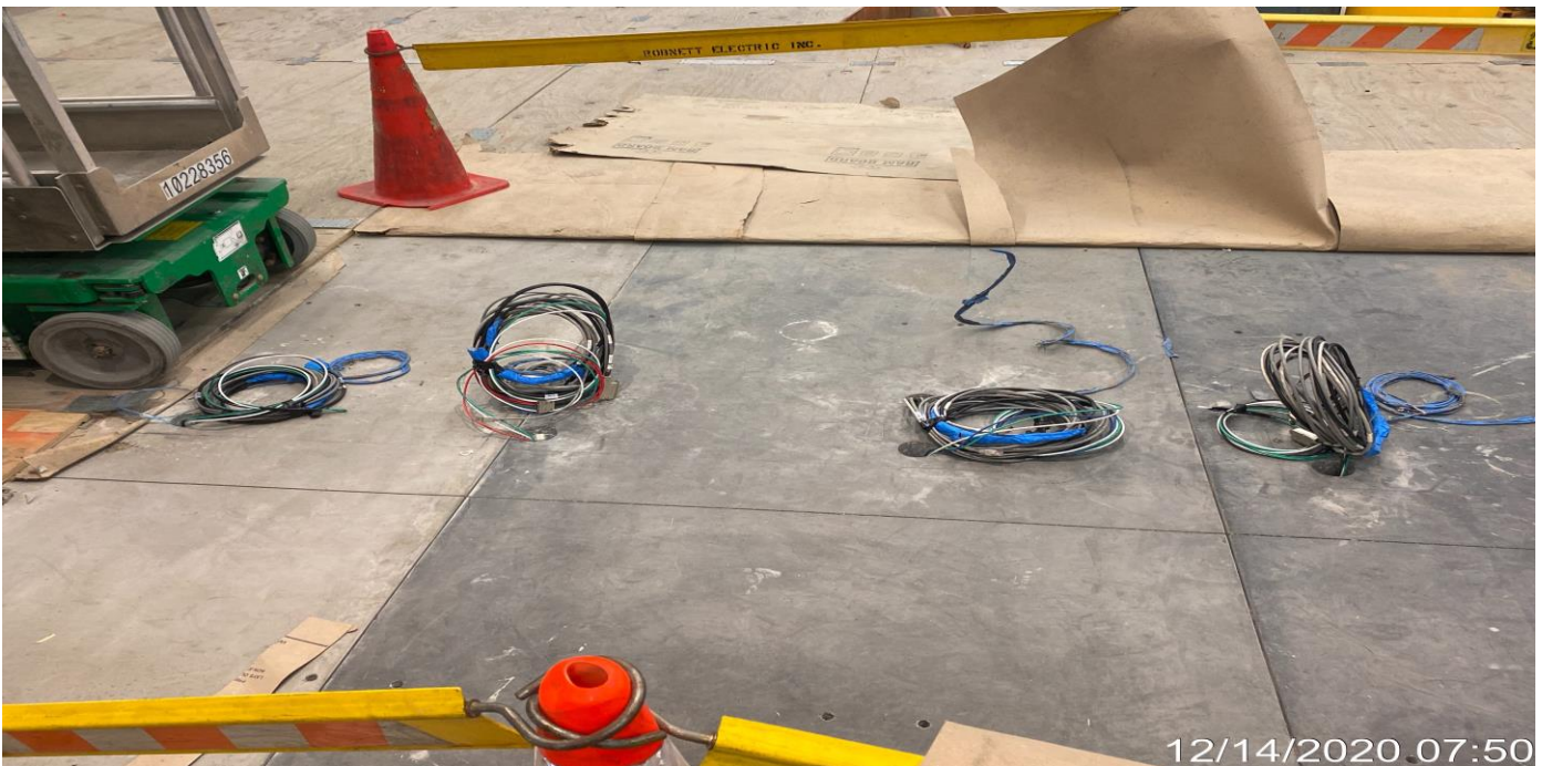
LEIMERT PARK STATION – Performing electrical work in preparation for the fare gate turnstile installation at the concourse Paid Area C-146.
