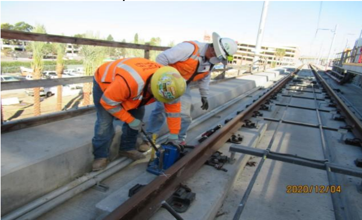
AVIATION/CENTURY- WSCC on Century/Aviation bridge SB track pull testing fastener 133 plinth 18 left side rail result was pass (looking northwest)
