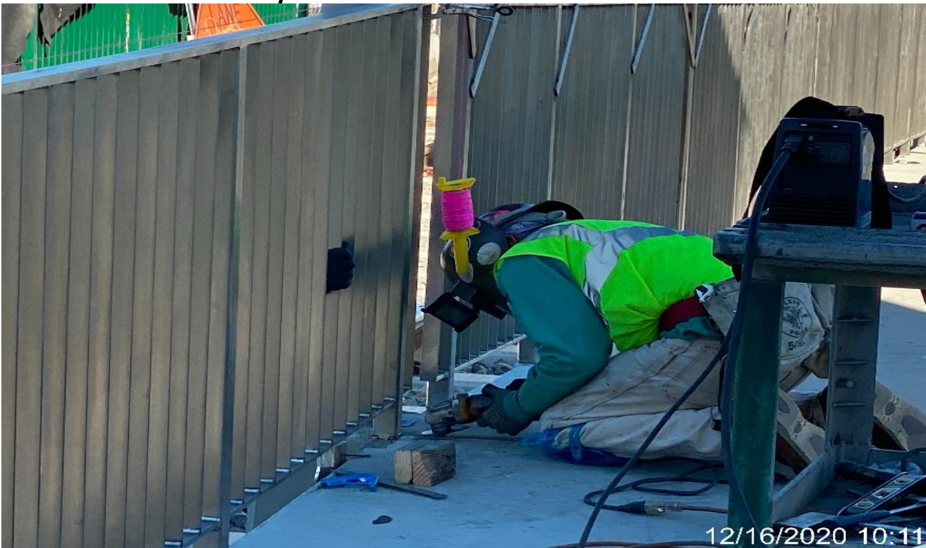
PARK MESA – Continue installing guardrails along the north and southbound side of the north end entrance ramp.
