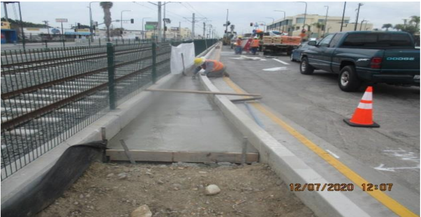
PARK MESA – Placing cobble mortar base to the southbound median curb of Crenshaw Blvd and 52nd St.
