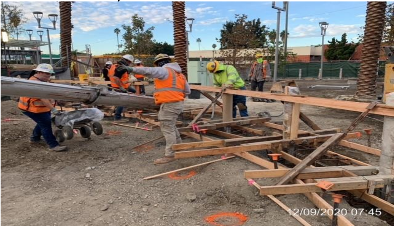
EXPO STATION – Placing concrete for the remaining steel bollards at the north end of the plaza.
