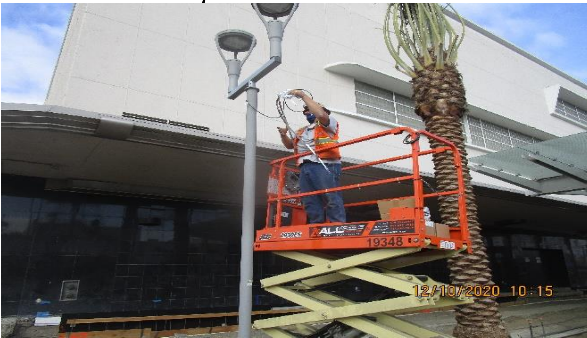
MLK STATION – Resume install AXIS T91L61 pole mount support brackets at pedestrian lighting
