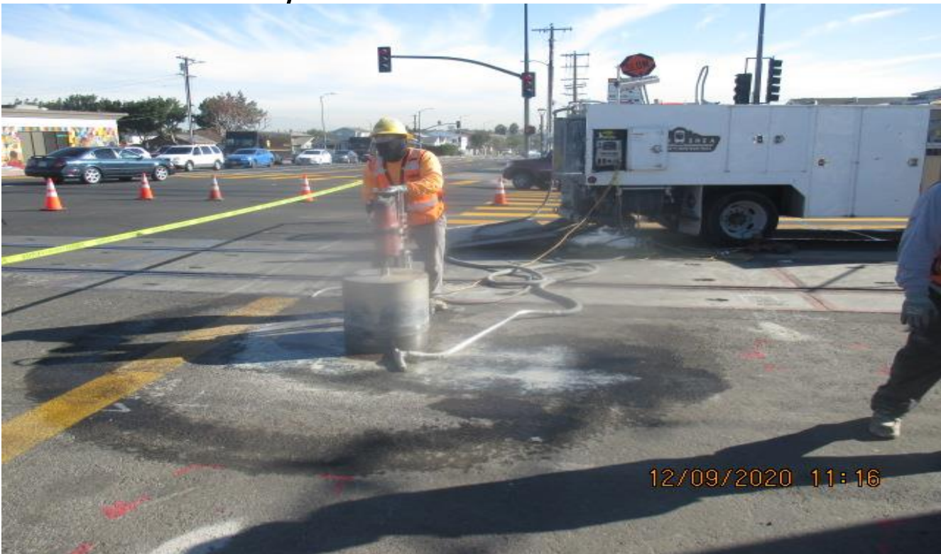
PARK MESA – Coring pavement in preparation of steel bollard installation on the crosswalk at Slauson Ave and Crenshaw Blvd.
