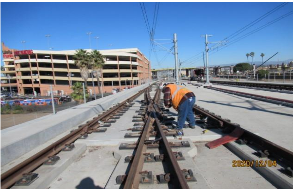
AVIATION/CENTURY- HCC working on open issues log Century/Aviation bridge 10K2LHXO SB track
