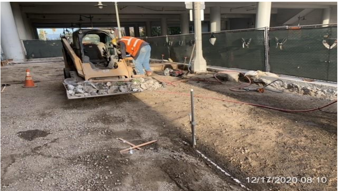
MLK STATION – Continue grading and compacting the far northwest area of the plaza.
