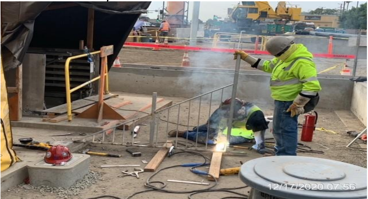
MLK STATION – Fabricating guardrails at the plaza to continue installation throughout Emergency Exit Stair South 2.
