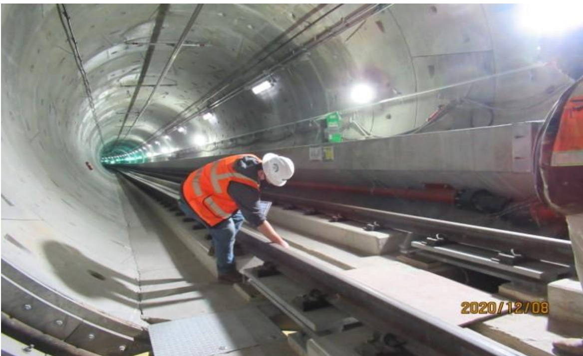
UG4 – WSCC field engineer logging non-conformance issues in UG4 NB track STA 401+55 (looking southwest).
