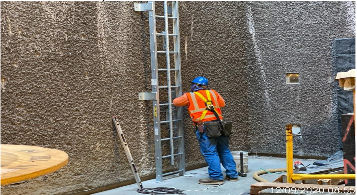
LEIMERT PARK STATION – Installing ladder inside the Emergency Ventilation Shaft North at the plaza.
