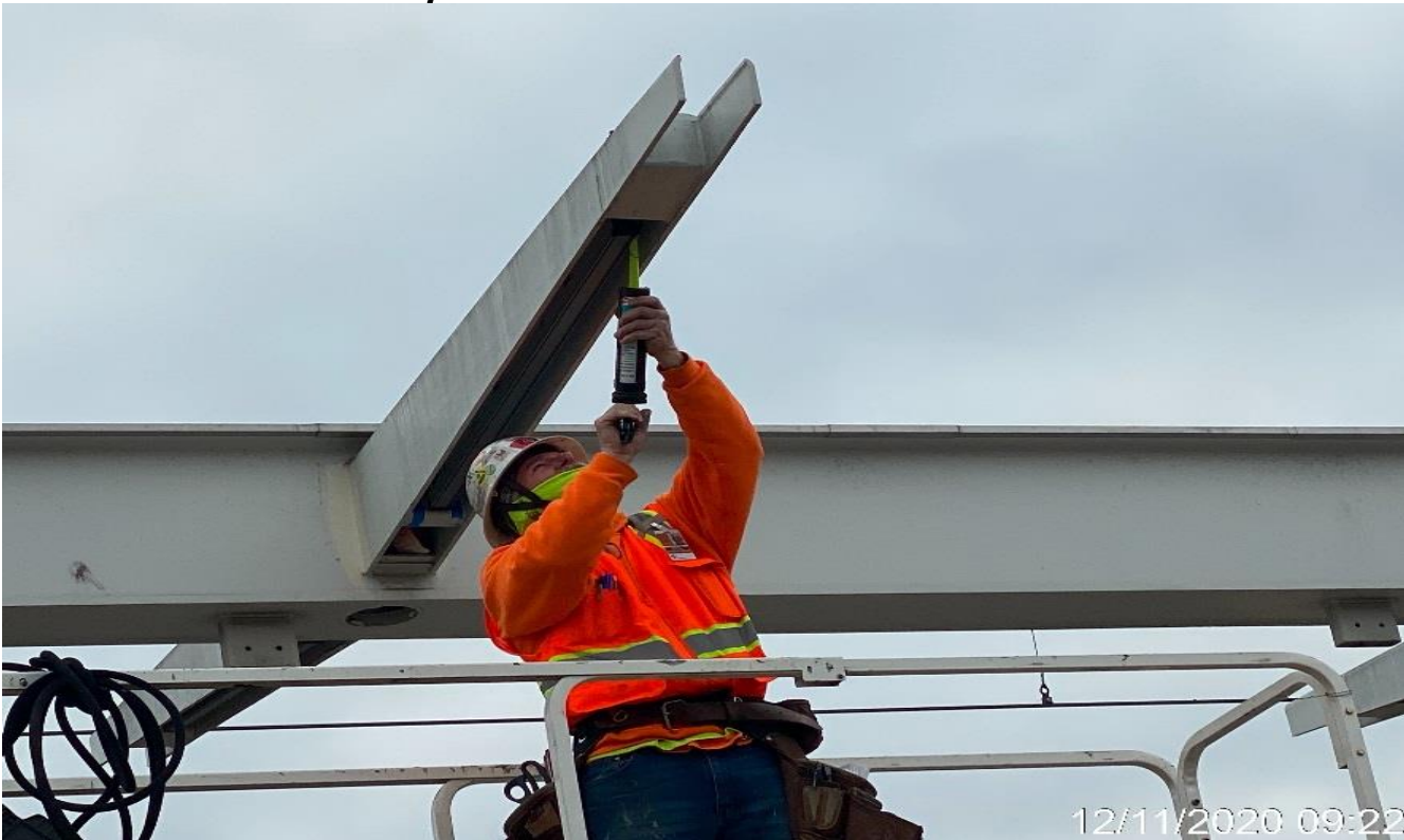
PARK MESA – Caulking and sealing BOCA light fixtures to the north end canopy outriggers at the platform.
