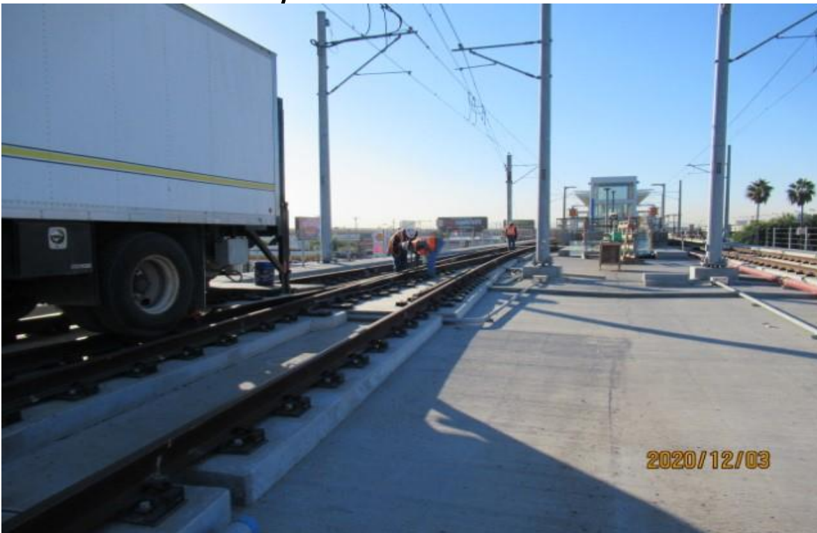
AVIATION/CENTURY- HCC working on open issues log at Century/Aviation bridge 10K1LHXO NB track (looking southeast) Rework
