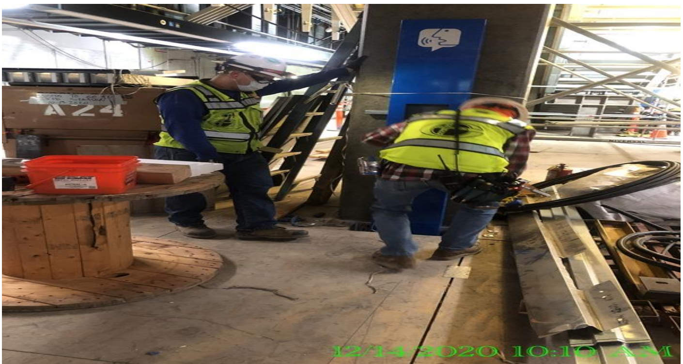
EXPO STATION – Drilled and anchored passenger telephone pedestal at the north end of the platform.
