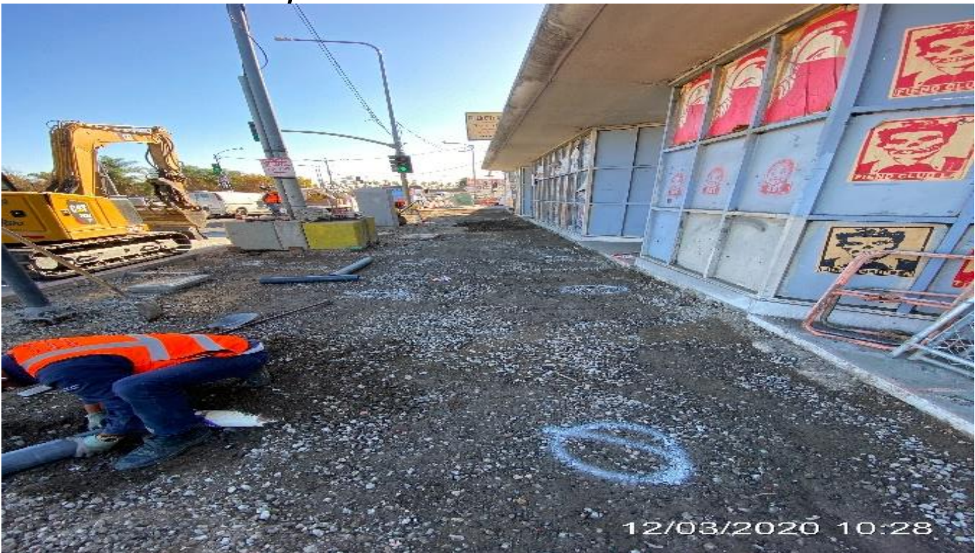
LEIMERT PARK STATION – Continue excavating/grading the entire sidewalk on southbound Crenshaw Blvd between Vernon Ave and Homeland Dr.
