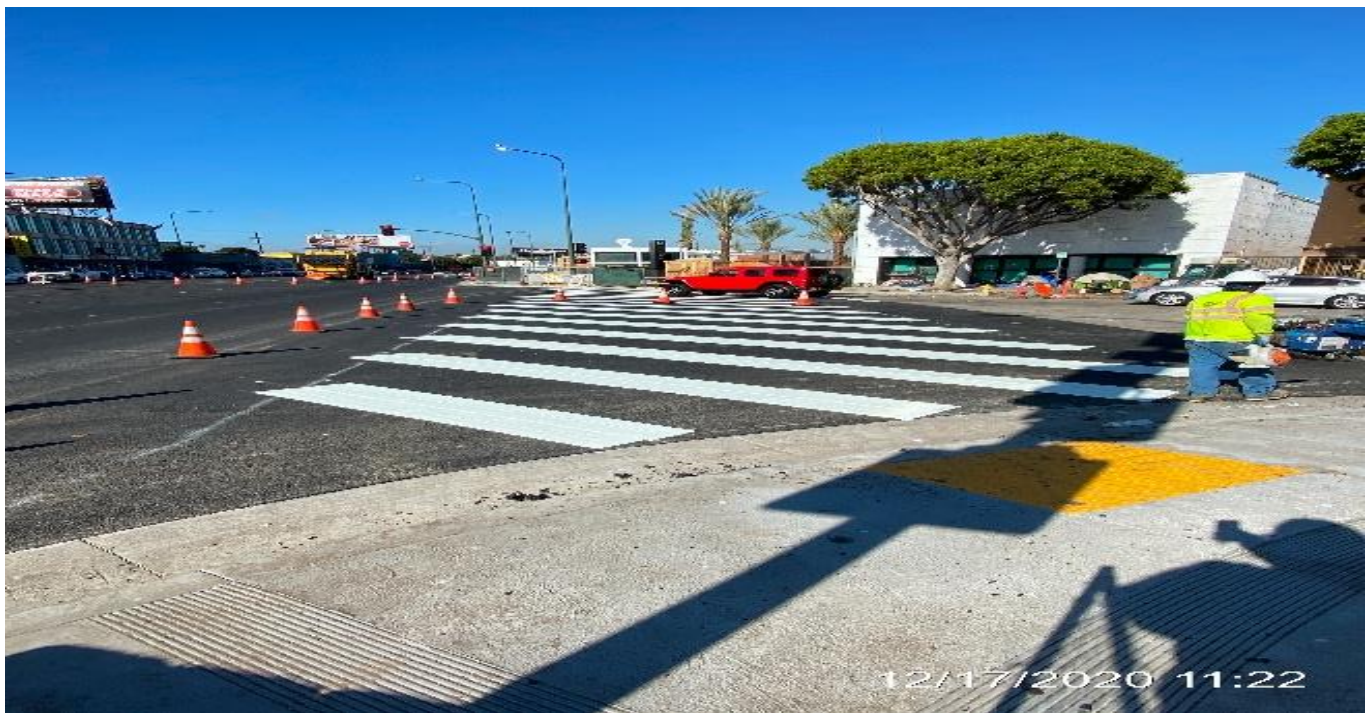
LEIMERT PARK STATION – Placing markings and lane striping along north and southbound Crenshaw Blvd from 48th St and ending at 43rd Pl.
