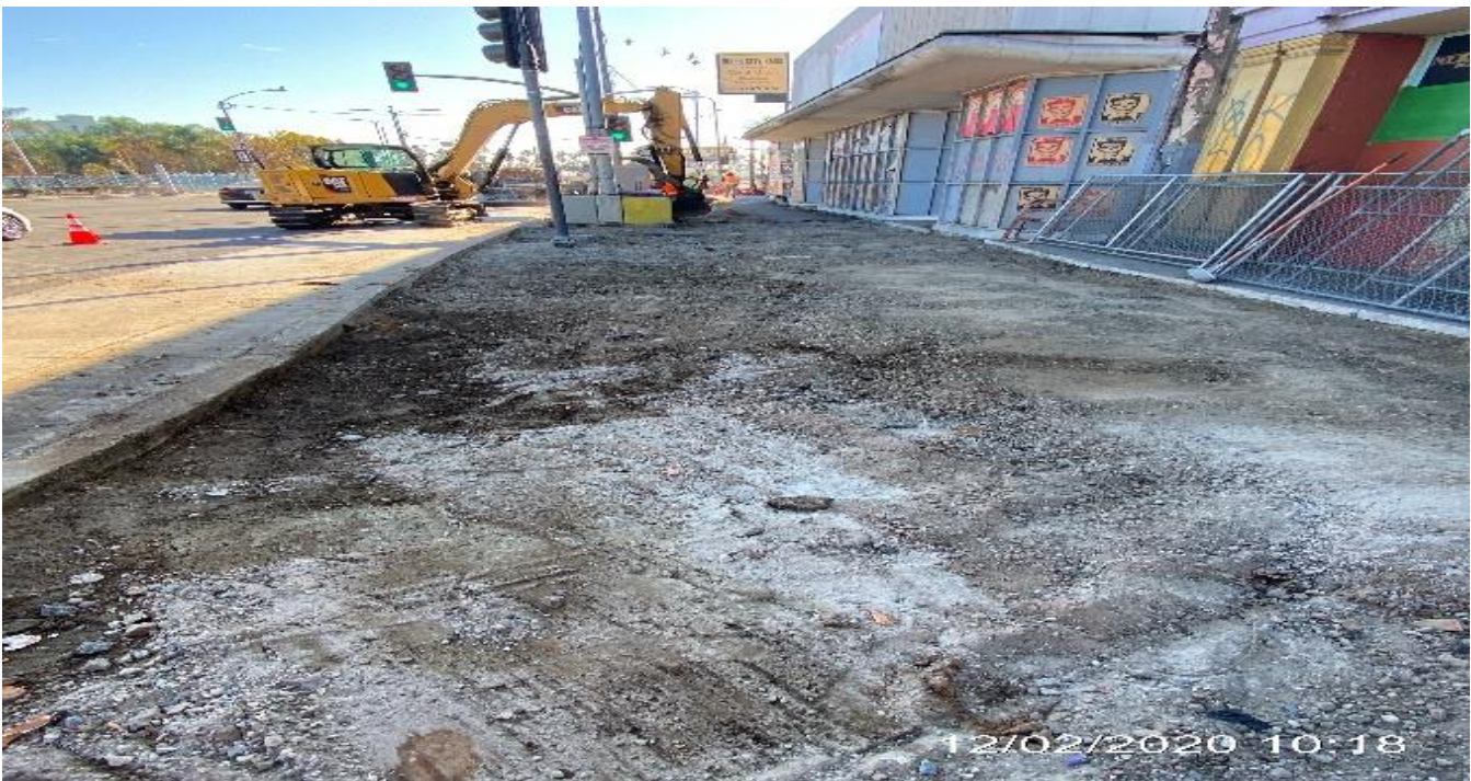
LEIMERT PARK STATION – Excavating/grading the entire sidewalk on southbound Crenshaw Blvd between Vernon Ave and Homeland Dr..
