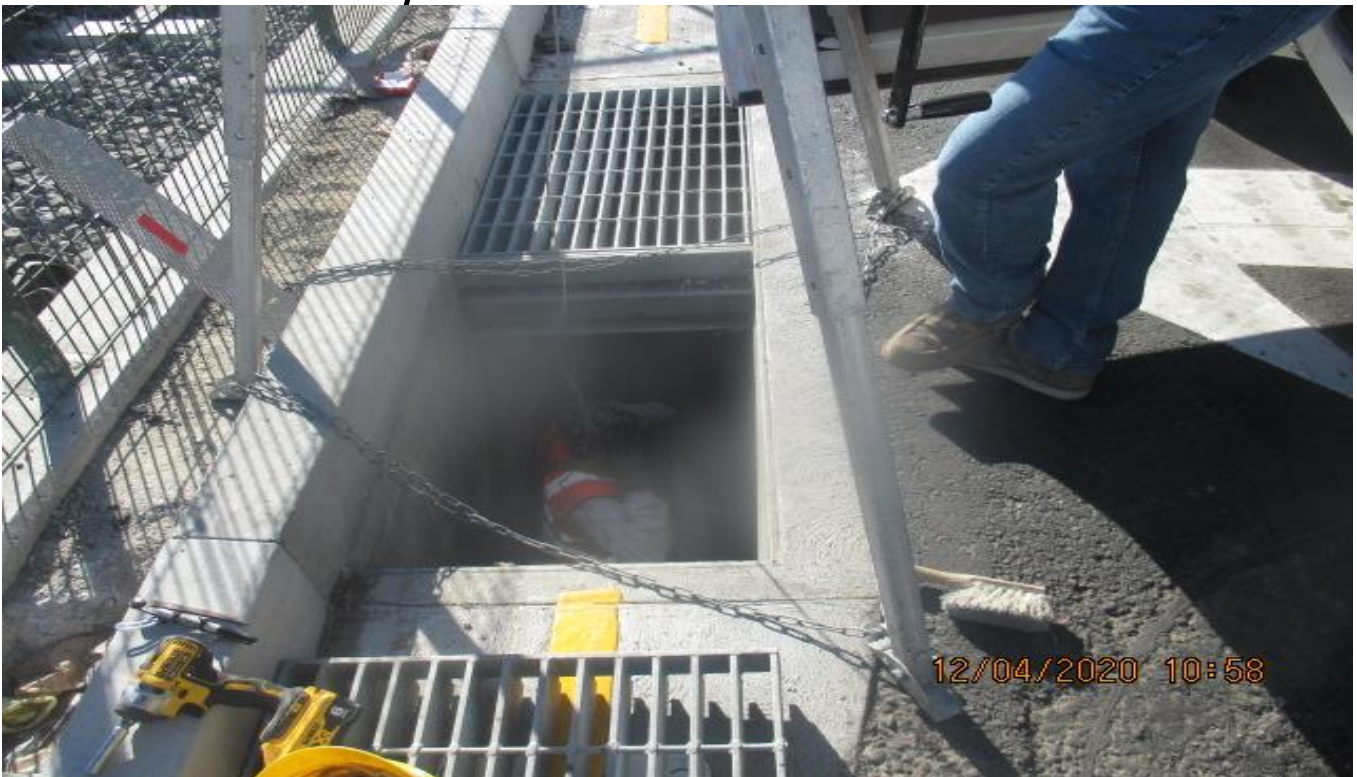
PARK MESA – Installing steel grates to Catch Basin #13 on southbound Crenshaw Blvd and Slauson Ave.
