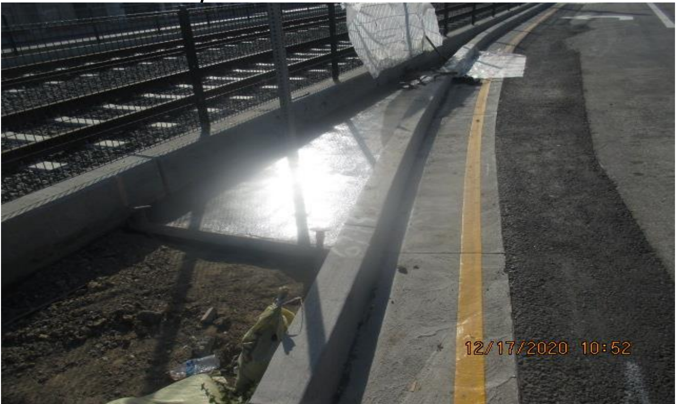
PARK MESA – Placing cobble mortar base to the southbound median curb of Crenshaw Blvd and 52nd St.
