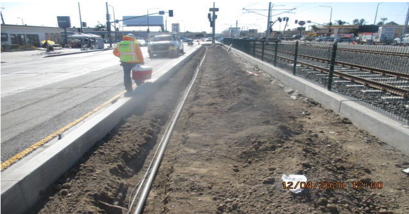
PARK MESA – Installing irrigation pipe line along the northbound median curb of Crenshaw Blvd and 48th St.
