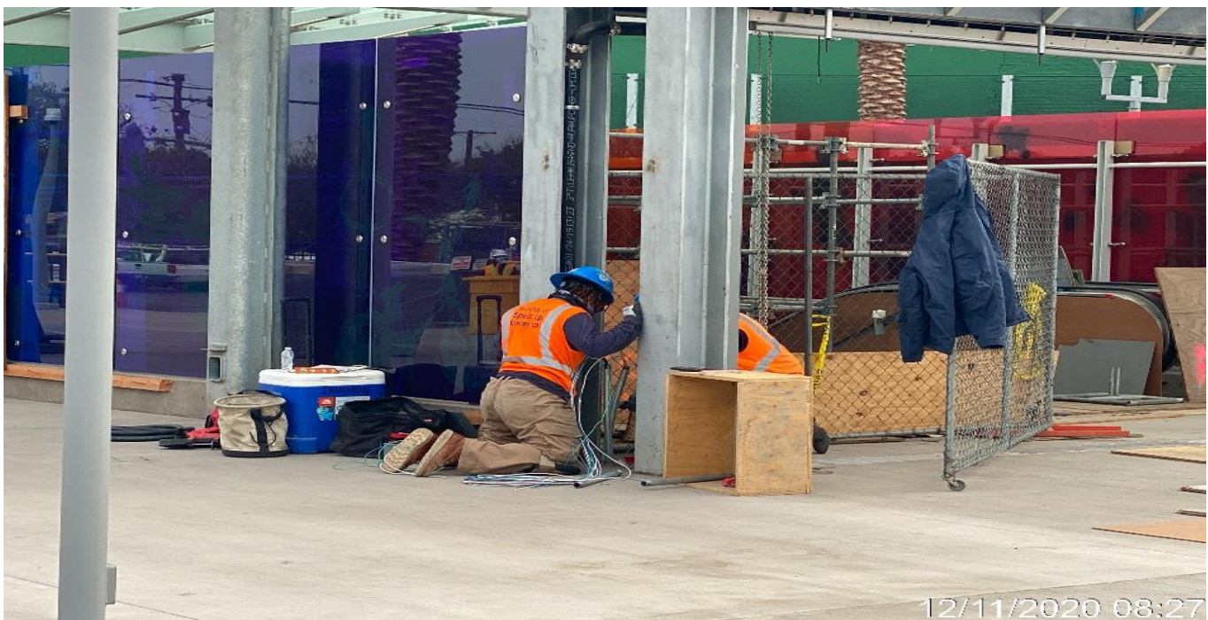
LEIMERT PARK STATION – Continue performing electrical work to the main entrance roll-up gate at the plaza.
