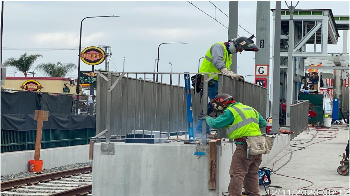
PARK MESA – Continue installing guardrails along the north and southbound side of the south end entrance ramp.
