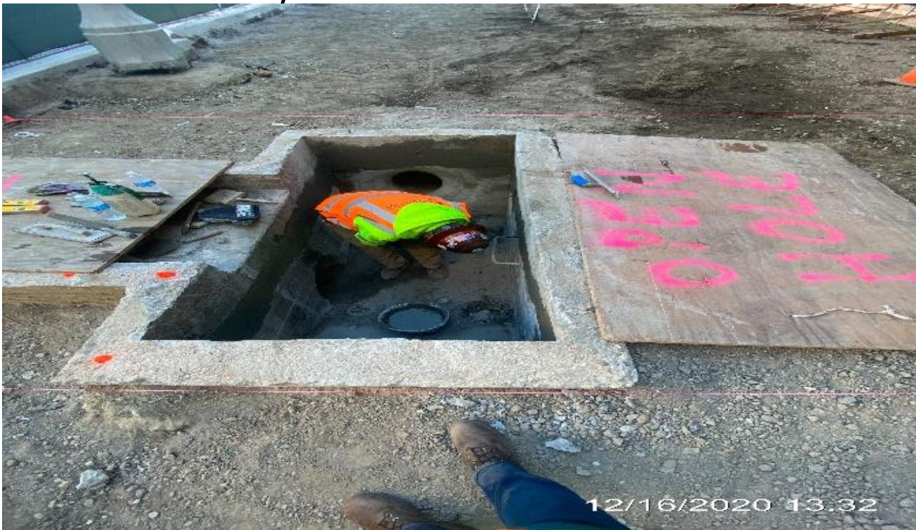
MLK STATION – Sacking and patching Catch Basin 3 on the northeast side of the plaza.
