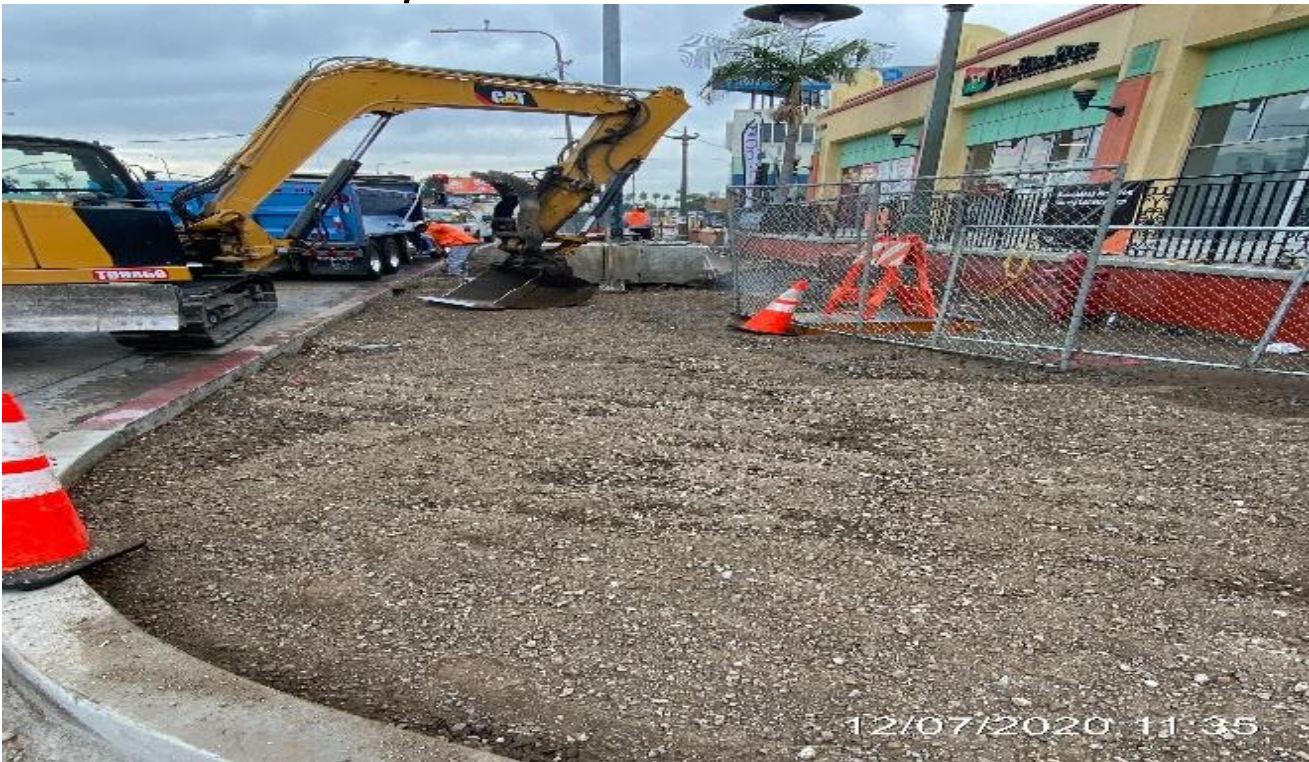
LEIMERT PARK STATION – Backfilling and compacting the entire sidewalk on southbound Crenshaw Blvd between Vernon Ave and Homeland Dr.
