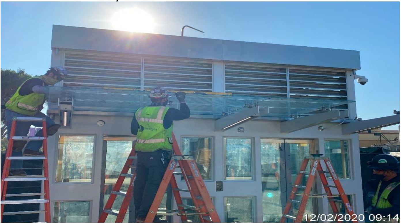
LEIMERT PARK STATION – Installing glass panels to the canopy outriggers of Elevators 1&2 at the plaza.
