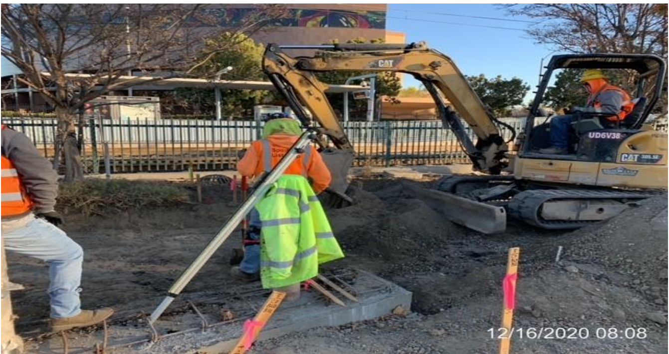
EXPO STATION - Continue grading/compacting and laying base at the northwest corner of the plaza.
