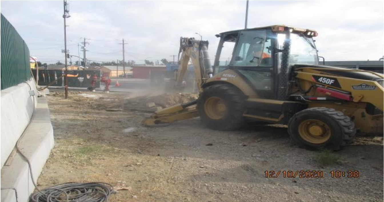
PARK MESA – Excavating/removing soil on eastbound New Road along the northbound barrier wall of UG3 in preparation for landscaping.
