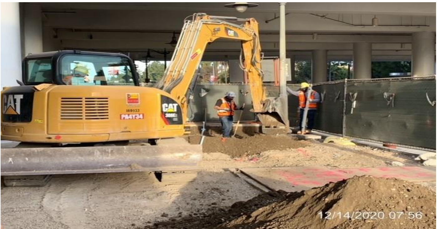
MLK STATION – Continue removing remaining sidewalk and grading the far northwest area of the plaza.
