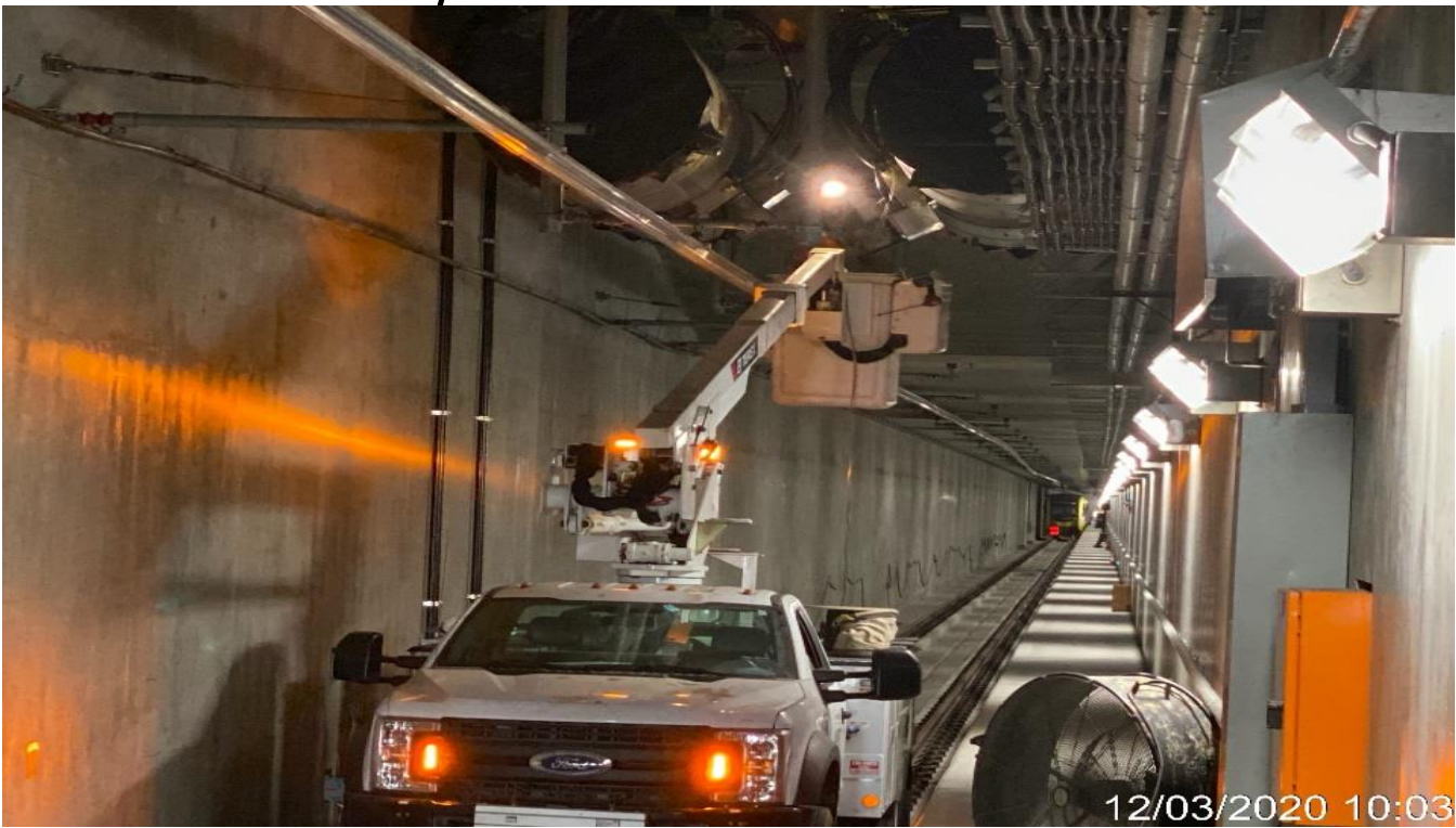
UG3 – Performing electrical work to the tunnel booster fans on the northbound tunnel.
