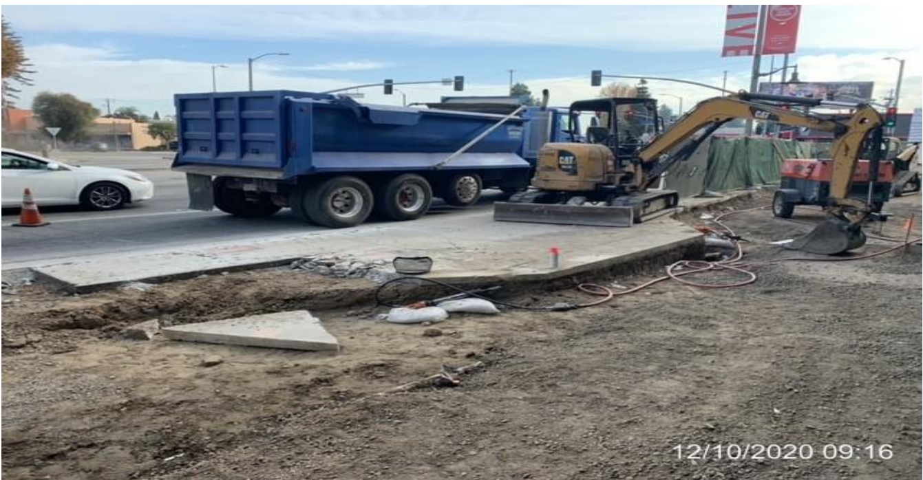
MLK STATION – Demolishing and removing remaining sidewalk sections at the far northwest area of the plaza.
