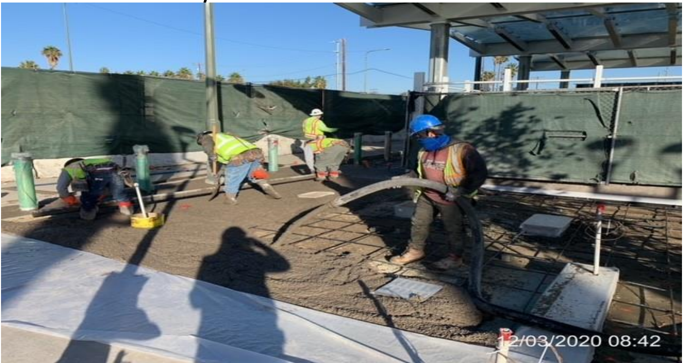
EXPO STATION SITE – Placing concrete for the architectural topping slab around the main entrance of the station.
