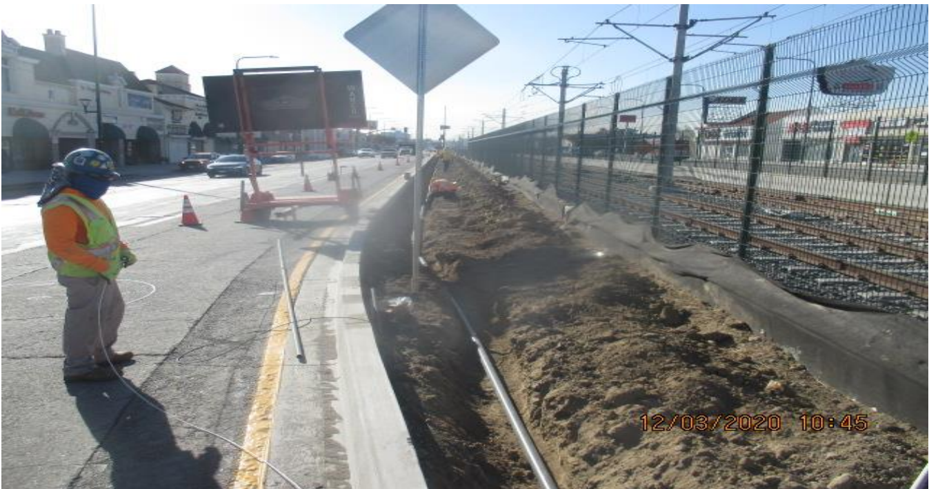
PARK MESA – Installing irrigation pipe line along the northbound median curb of Crenshaw Blvd on 57th St and moving toward 54th St.
