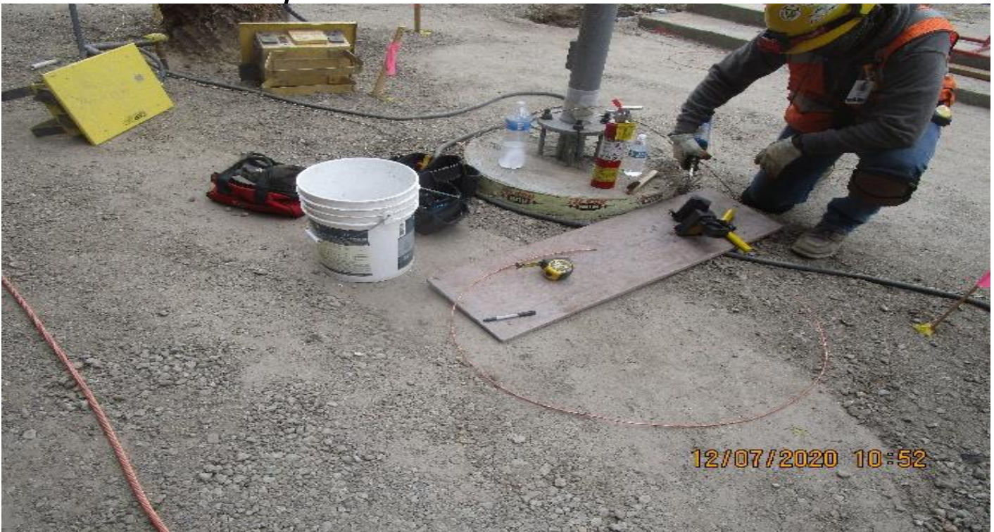
MLK STATION – Continue installing ground grid system at the north end section of the plaza.
