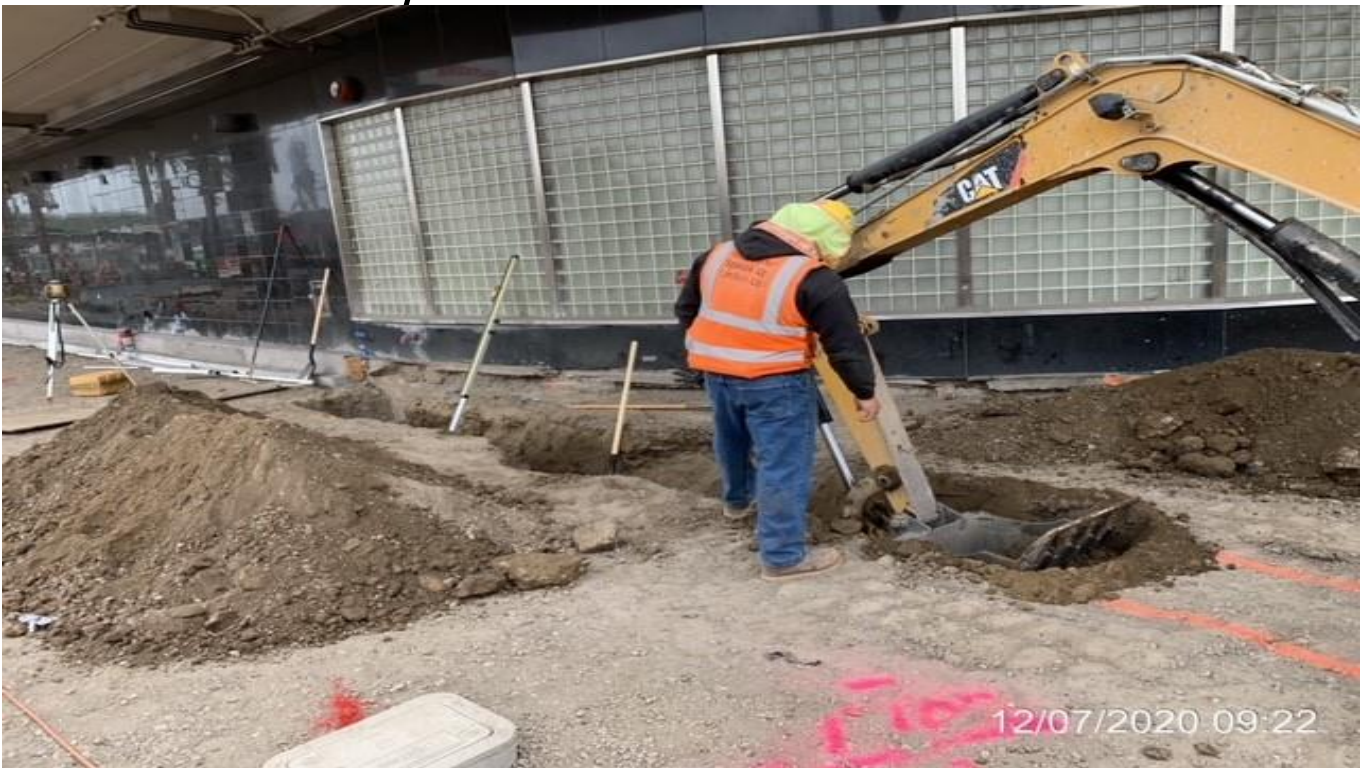
MLK STATION – Excavating/trenching for the Capri gas line installation at the north side of the plaza.
