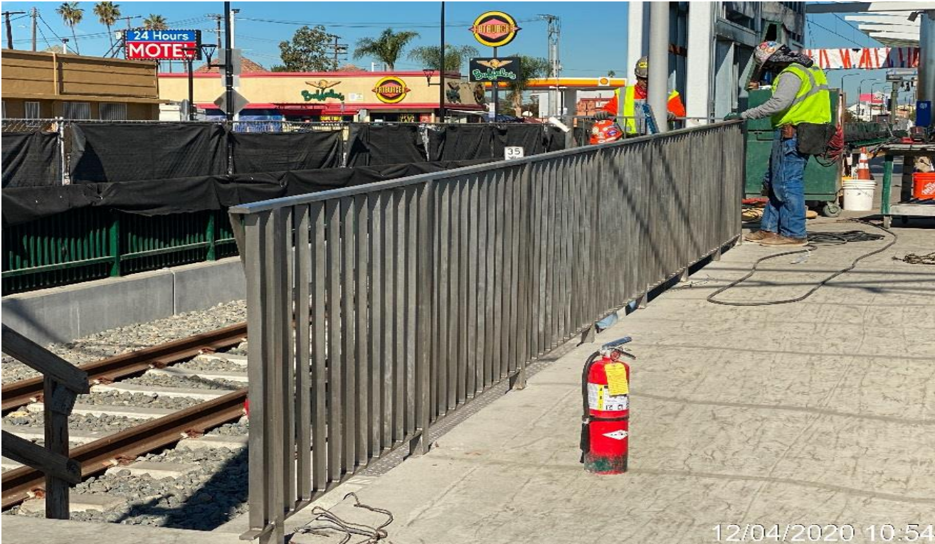
PARK MESA – Installing guardrails along the southbound side of the south end entrance ramp.
