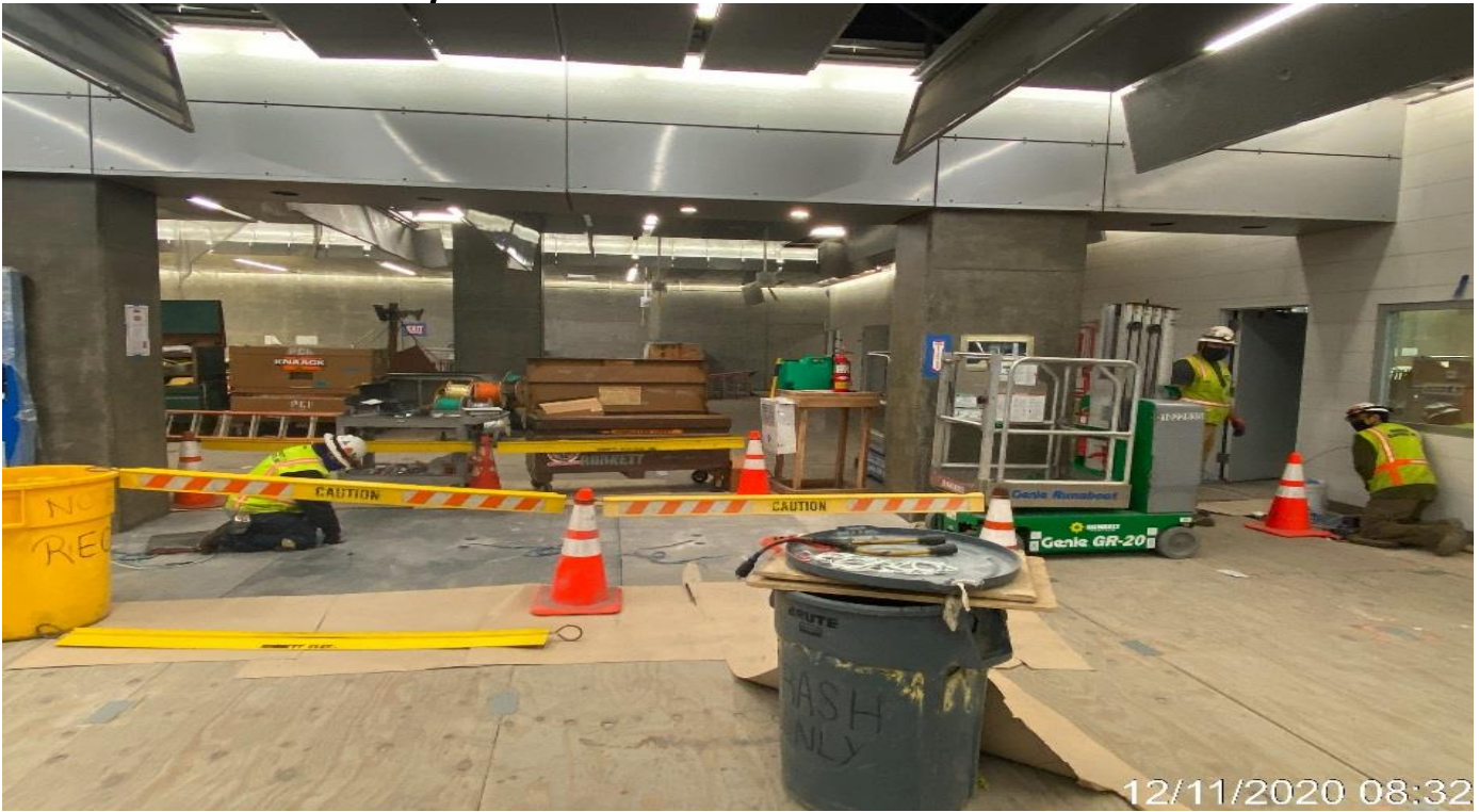
LEIMERT PARK STATION – Performing electrical work in preparation for the fare gate turnstile installation at the concourse Paid Area C-146.
