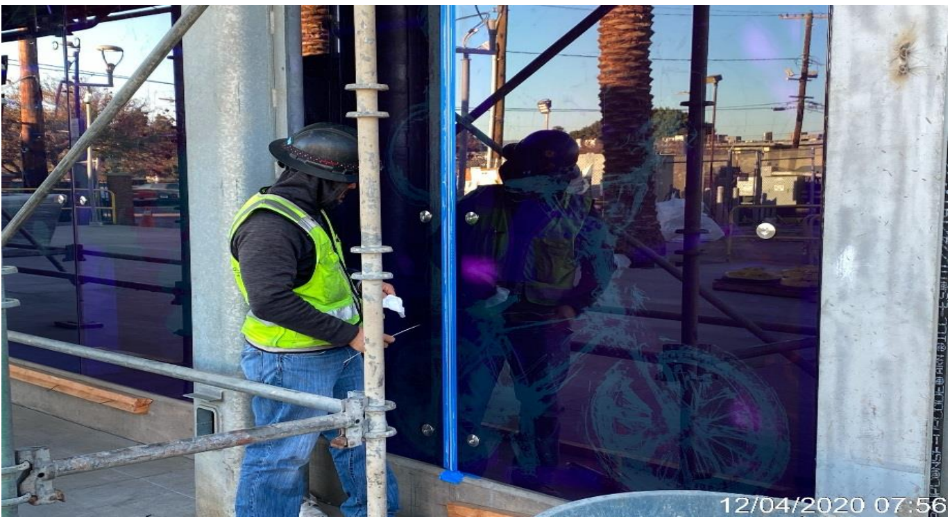
LEIMERT PARK STATION – Caulking and sealing the art glass around the main entrance canopy at the plaza.
