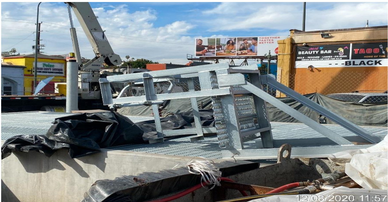
LEIMERT PARK STATION – Preparing to install ladder inside the Emergency Ventilation Shaft North at the plaza.
