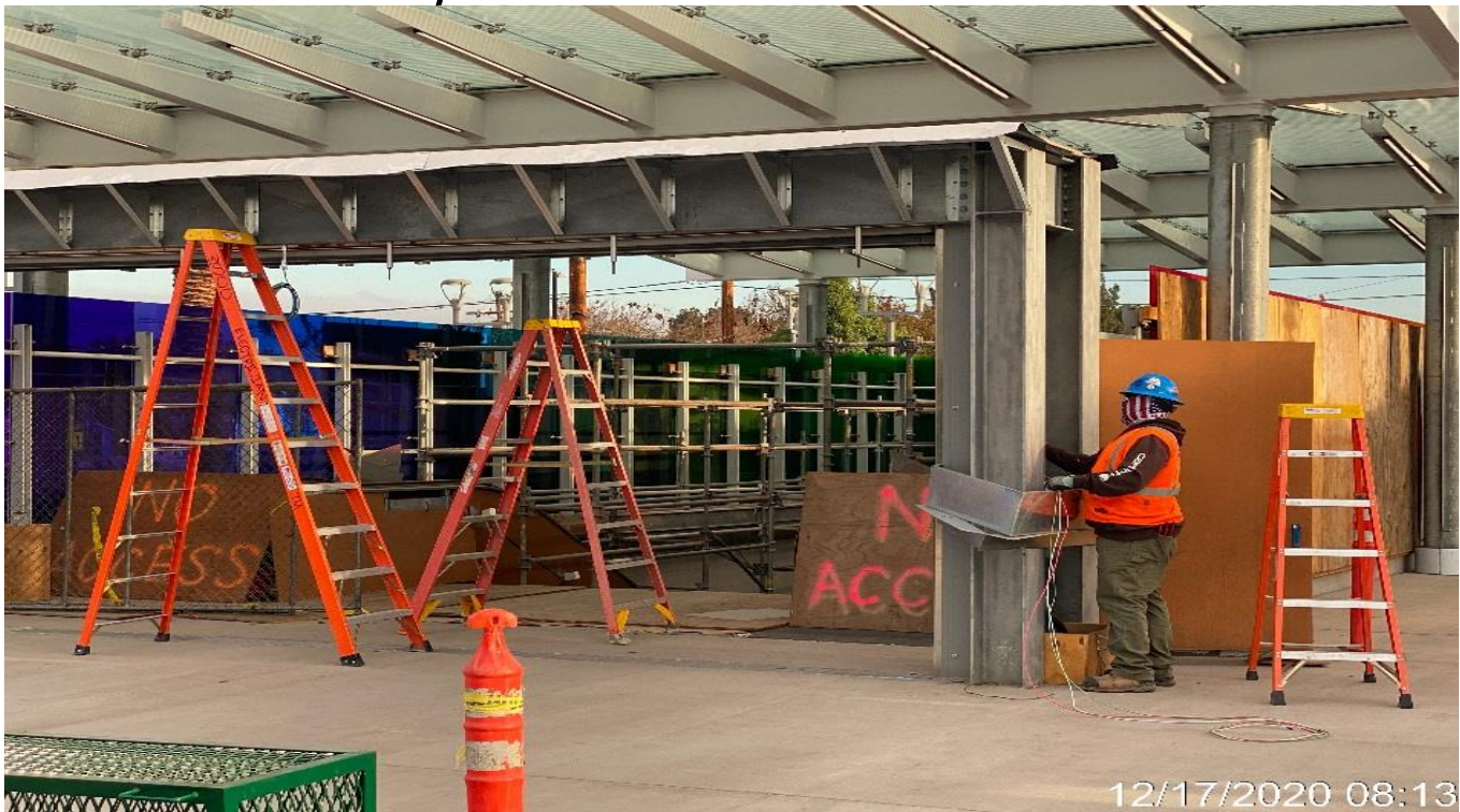
LEIMERT PARK STATION – Continue performing electrical work to the main entrance roll-up gate at the plaza.
