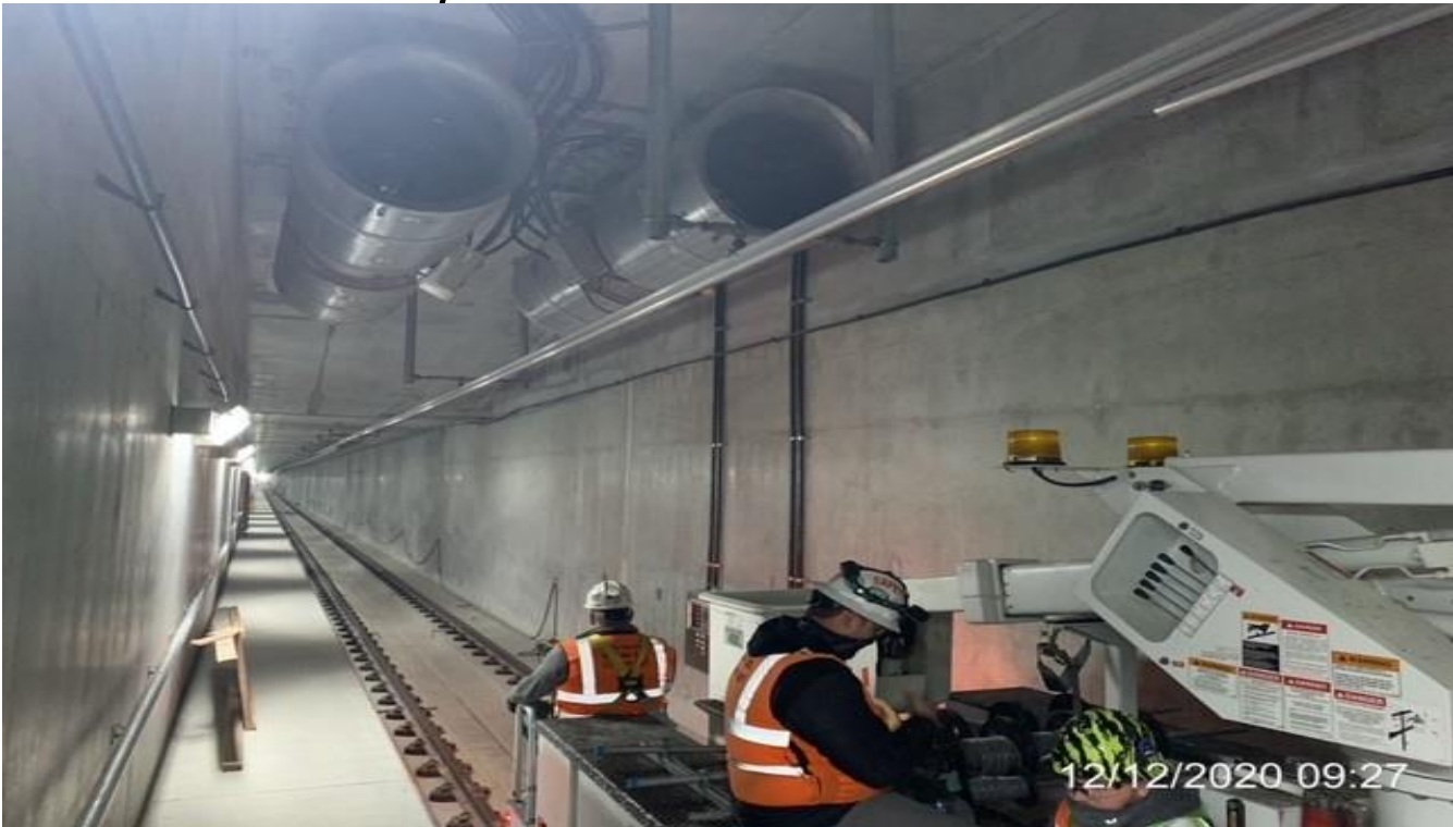
UG3 – Performing mechanical testing to the tunnel booster fans on the southbound tunnel.
