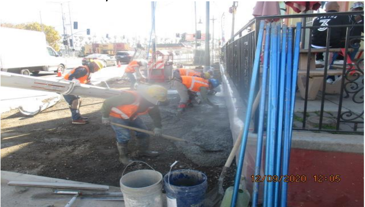
LEIMERT PARK STATION – Placing concrete for the entire sidewalk on southbound Crenshaw Blvd between 43rd Pl and Vernon Ave.
