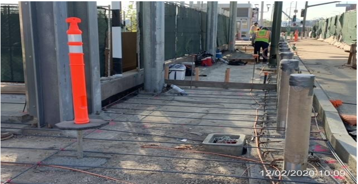
EXPO STATION – Building formwork and placing rebar for the architectural topping slab around the main entrance of the station.
