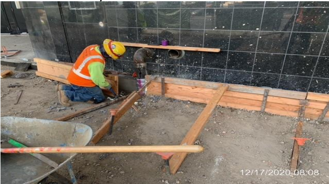
MLK STATION – Continue expansion board installation along the north side curb of the Mall at the plaza.
