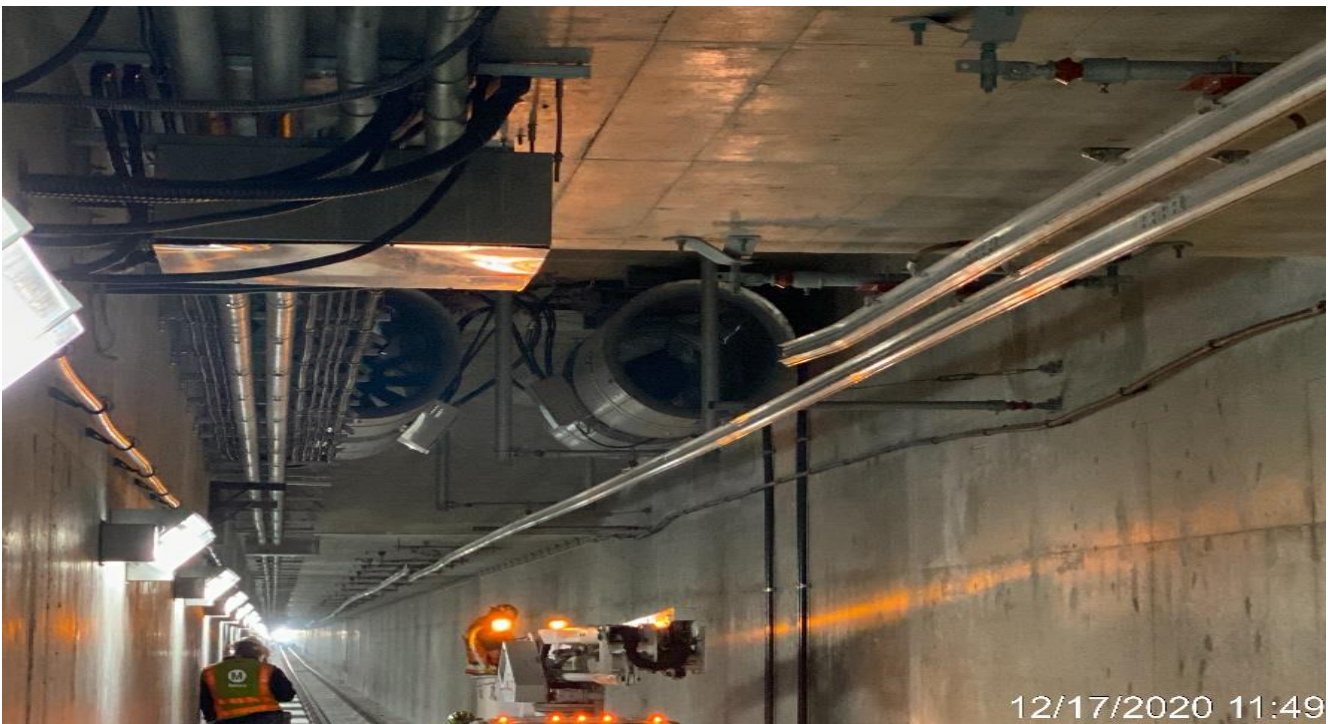
UG3 – Performing pre-start up inspections to the tunnel booster fans on the northbound tunnel.
