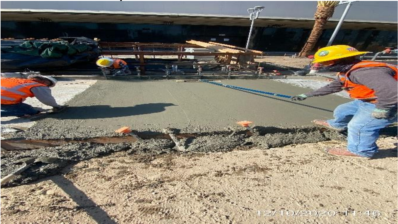
MLK STATION – Built formwork and placed concrete for bus pad along the east side of the plaza.
