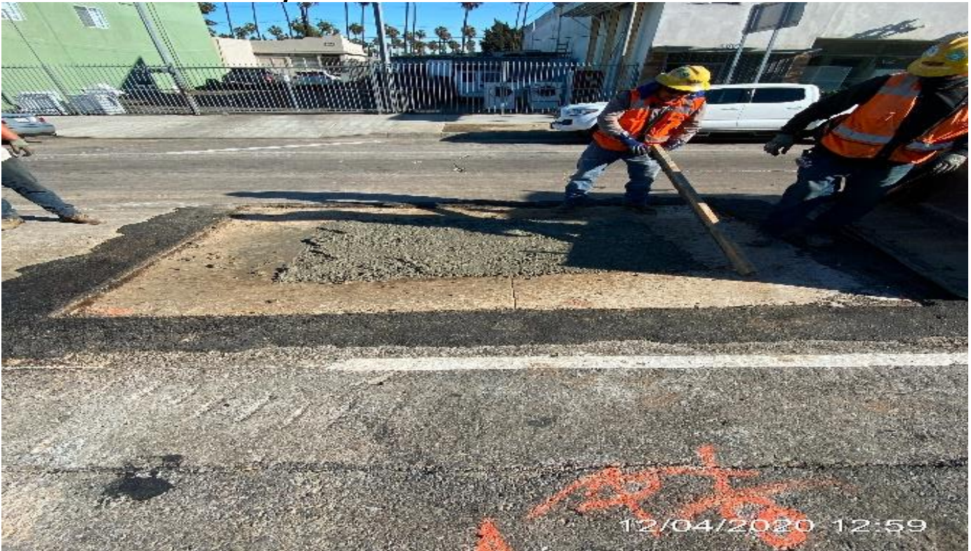
PARK MESA – Placing concrete over existing overhead sign foundation on northbound Crenshaw Blvd and 48th St.
