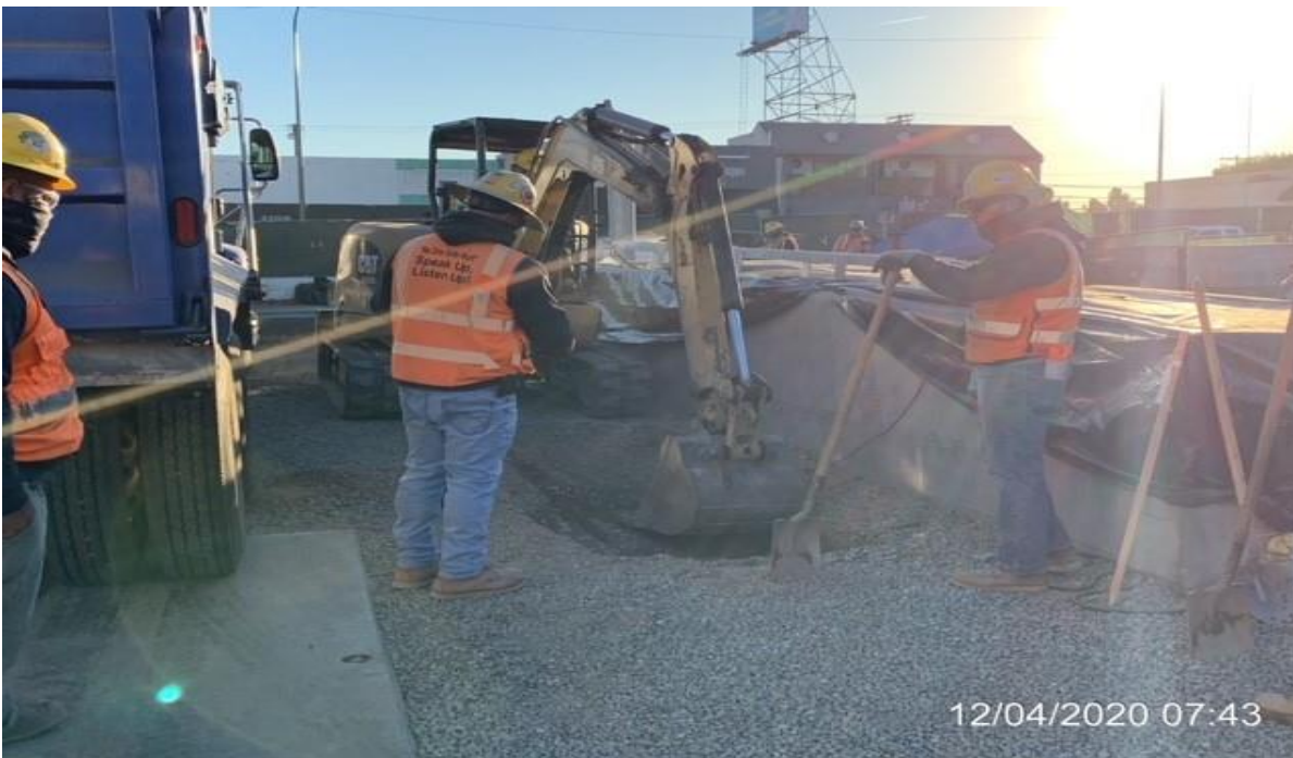
EXPO STATION– WSCC crew excavating for curb and gutter of service road.
