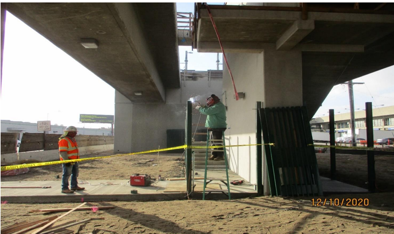
AVIATION/CENTURY- Welding on the fence gate at the SW corner of Aviation and Century.
