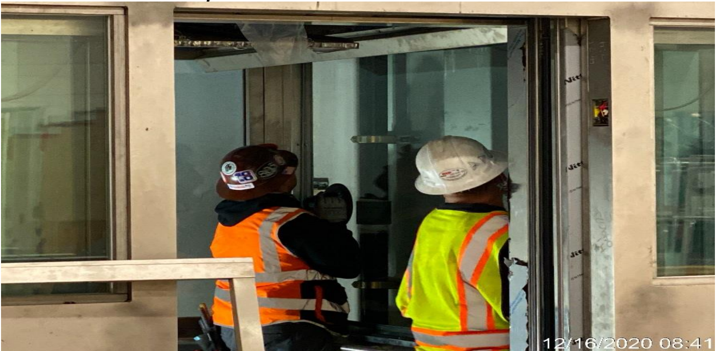
LEIMERT PARK STATION – Installing glass panels inside all 4 Elevator cabs at the concourse level.
