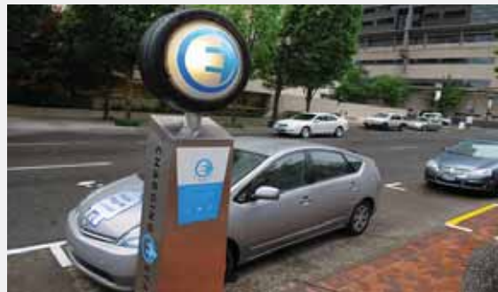
Curbside electric Vehicle charging station, Portland, OR
