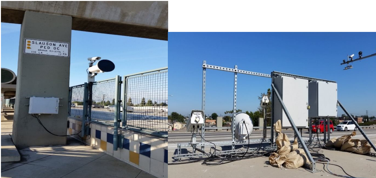
Figure 17: Photo of VPDS Camera and Equipment
