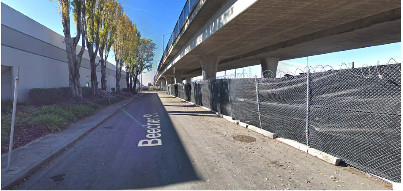
Figure 4. - Extensive viaduct structure will provide additional widths for the frontage roads but also introduce “eye sores” to neighborhood.
