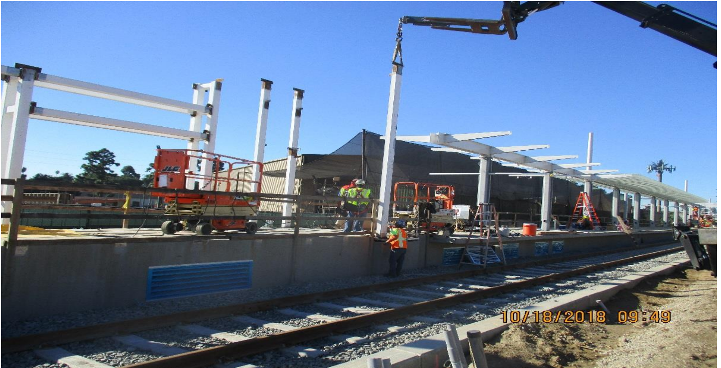
WEST STATION - Erecting the east ticket fare gate at the West Station.
