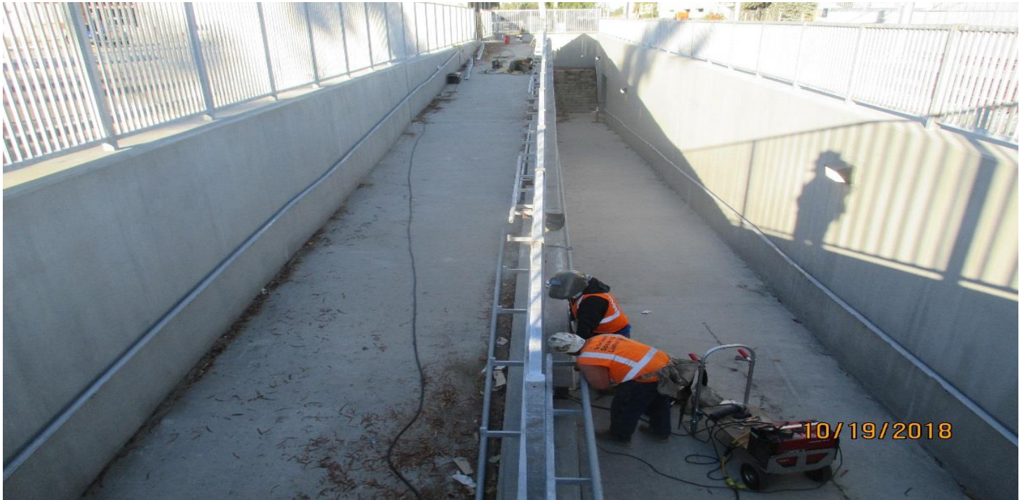
(AG-7) FCBC PED UP- Erecting the hand rails for the FCBC NB side walkway.
