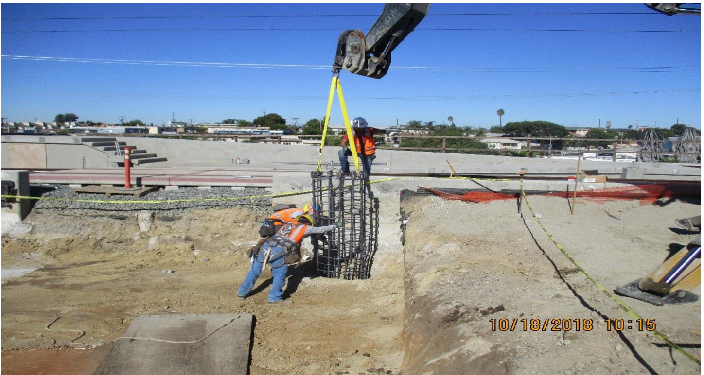
DOWNTOWN INGLEWOOD STATION- Placing CIDH rebar cage at the Inglewood Station east fare gate.
