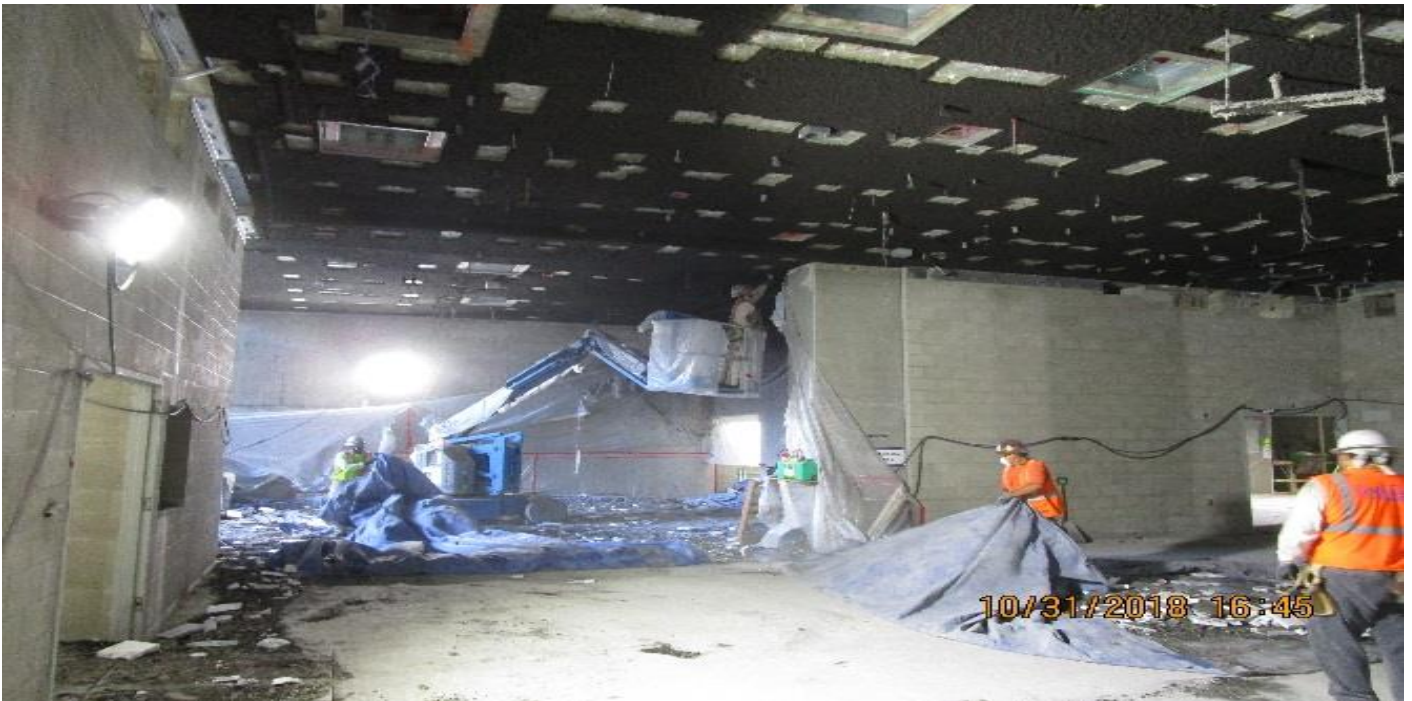
EXPOSITION/CRENSHAW STATION – Installation of acoustical spray at the ceiling in the Public Area at concourse.
