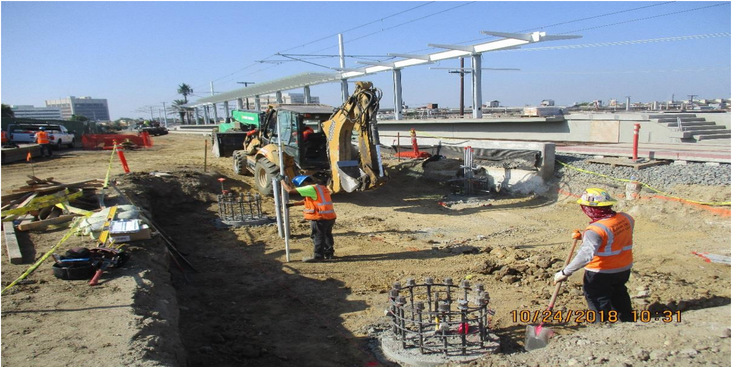
DOWNTOWN INGLEWOOD STATION- Grading for grade beam and slab at the Inglewood Station east fare gate.
