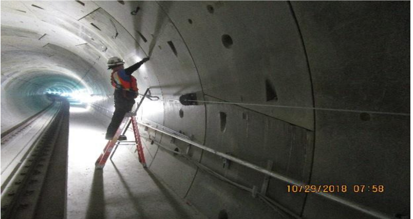
TUNNEL – Installation of F5 lighting fixtures in the NB tunnel between MLK and Vernon Stations.
