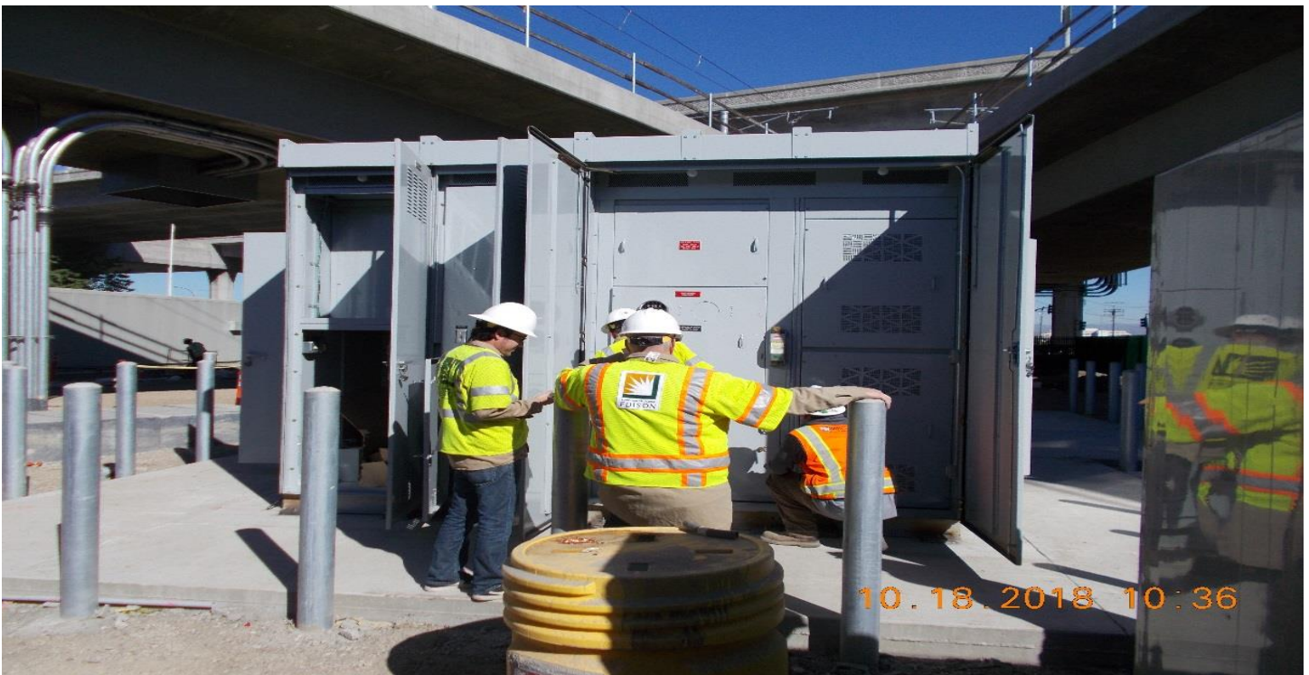
TPSS- TPSS #1- SCE was inspecting their metering gear.
