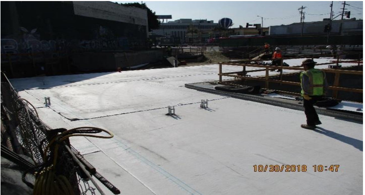
LEIMERT PARK STATION – Installation of waterproofing at the roof east of the Entrance Structure.
