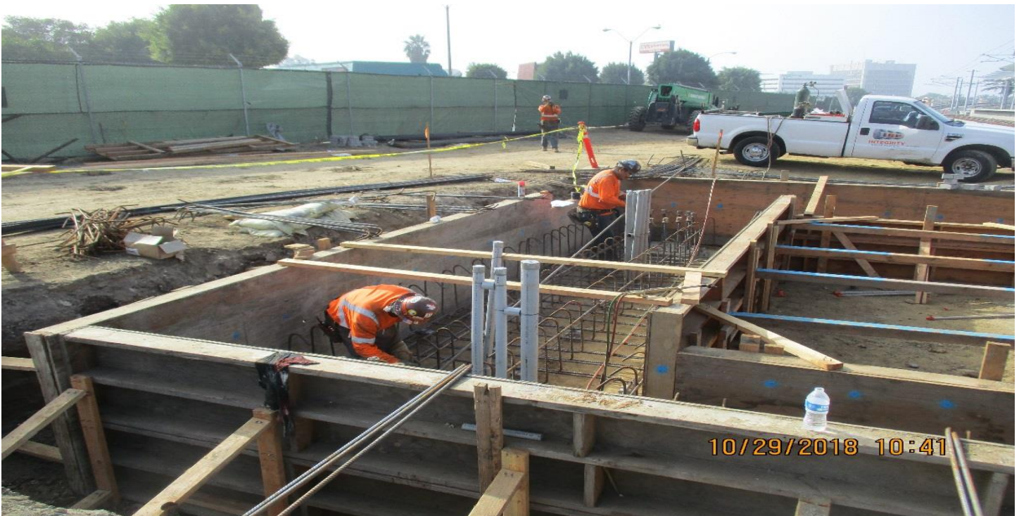
DOWNTOWN INGLEWOOD STATION - Installing rebar at the Inglewood Station east fare gate.
