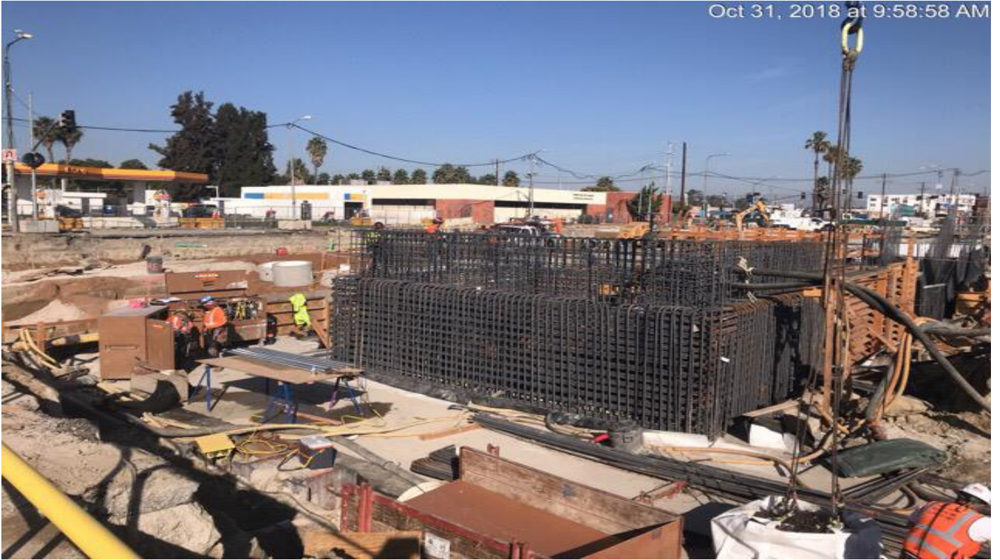
EXPOSITION/CRENSHAW STATION – Installation of rebar for wall R7 at the plaza level.
