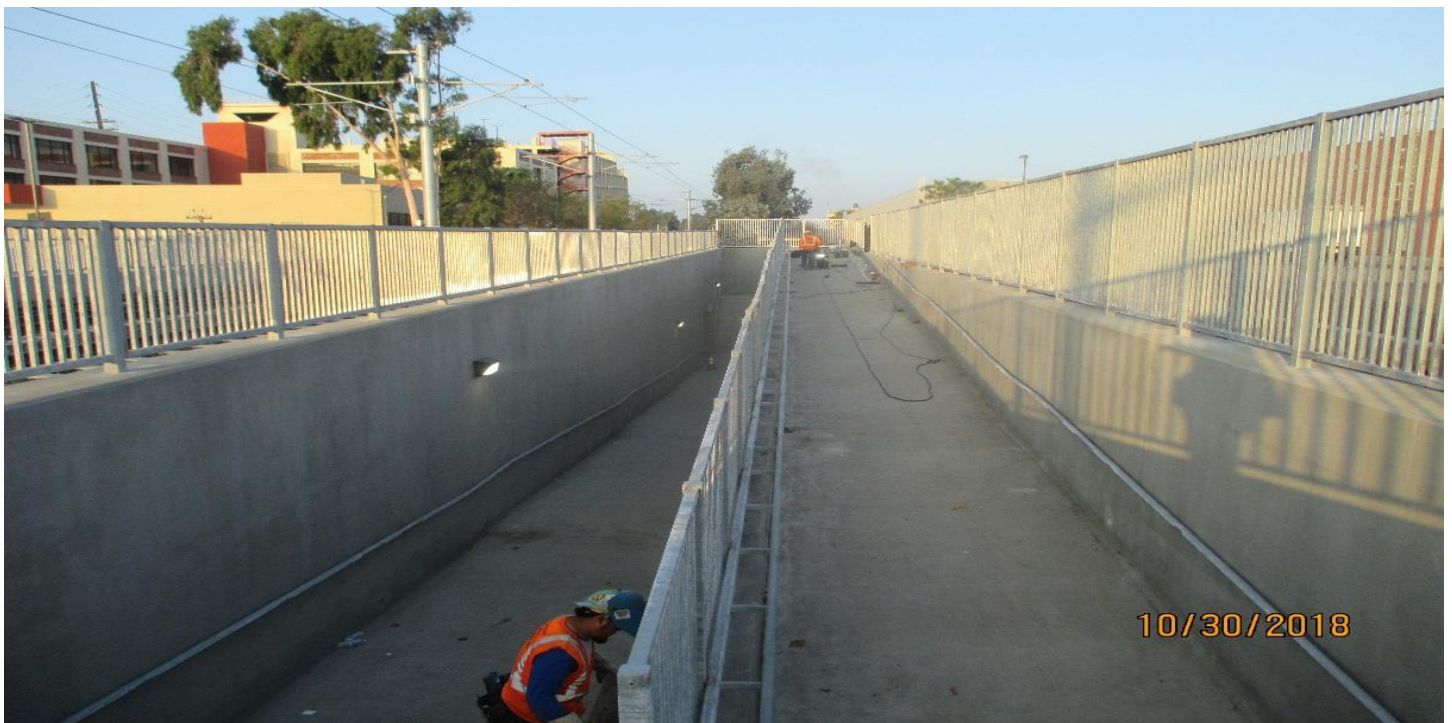
(AG-7) FCBC PED UP- Hand rail erection for the SB side of the FCBC walkway underpass.
