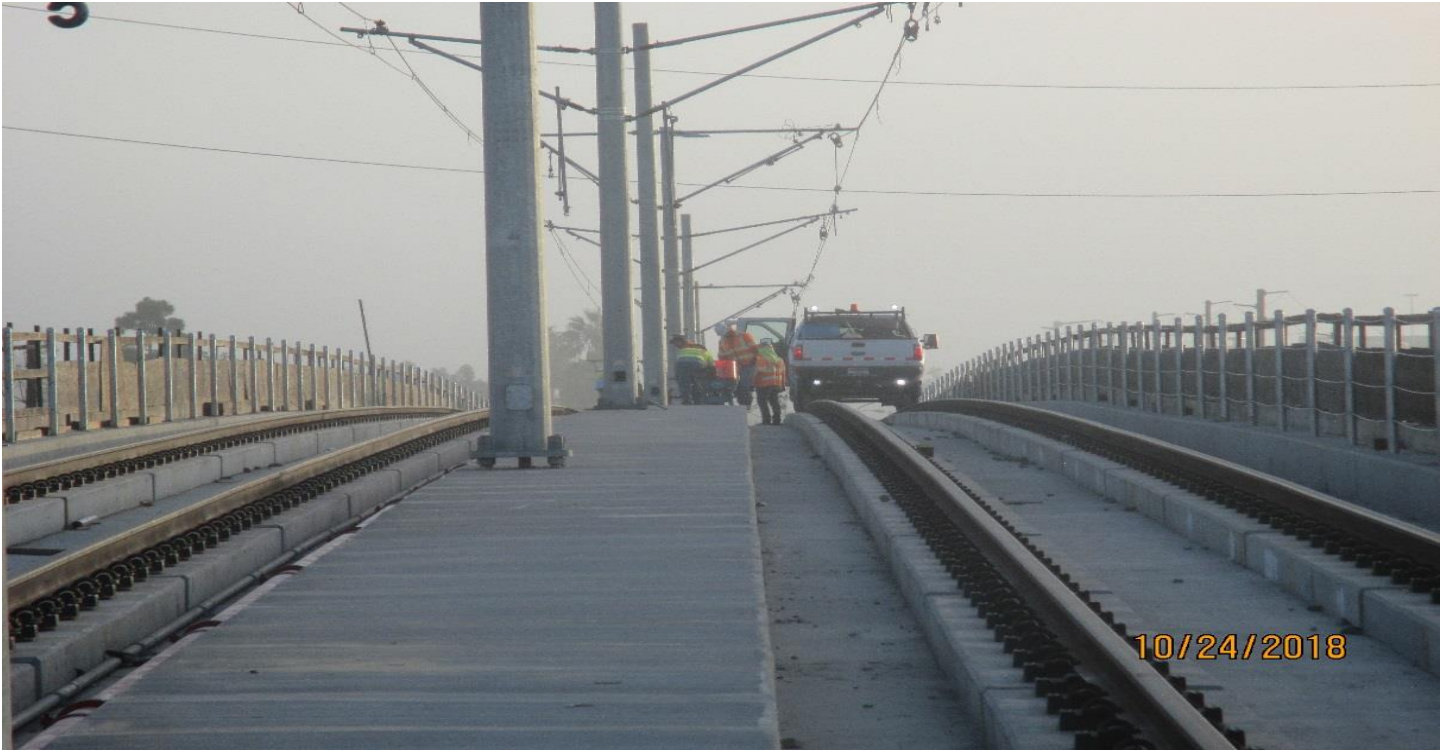
(AG-5) I-405 BRIDGE- Stringing cable for the cable rail fence on the 405 Bridge.
