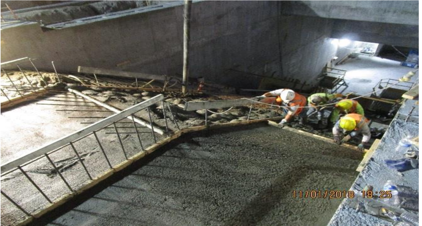
EXPOSITION/CRENSHAW STATION – Concrete placement for the sloped deck section Y-3 at the Entrance Structure.
