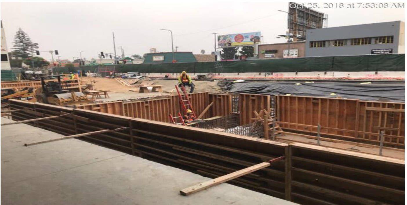
MARTIN LUTHER KING JR. STATION- Installation of formwork for the plaza walls.
