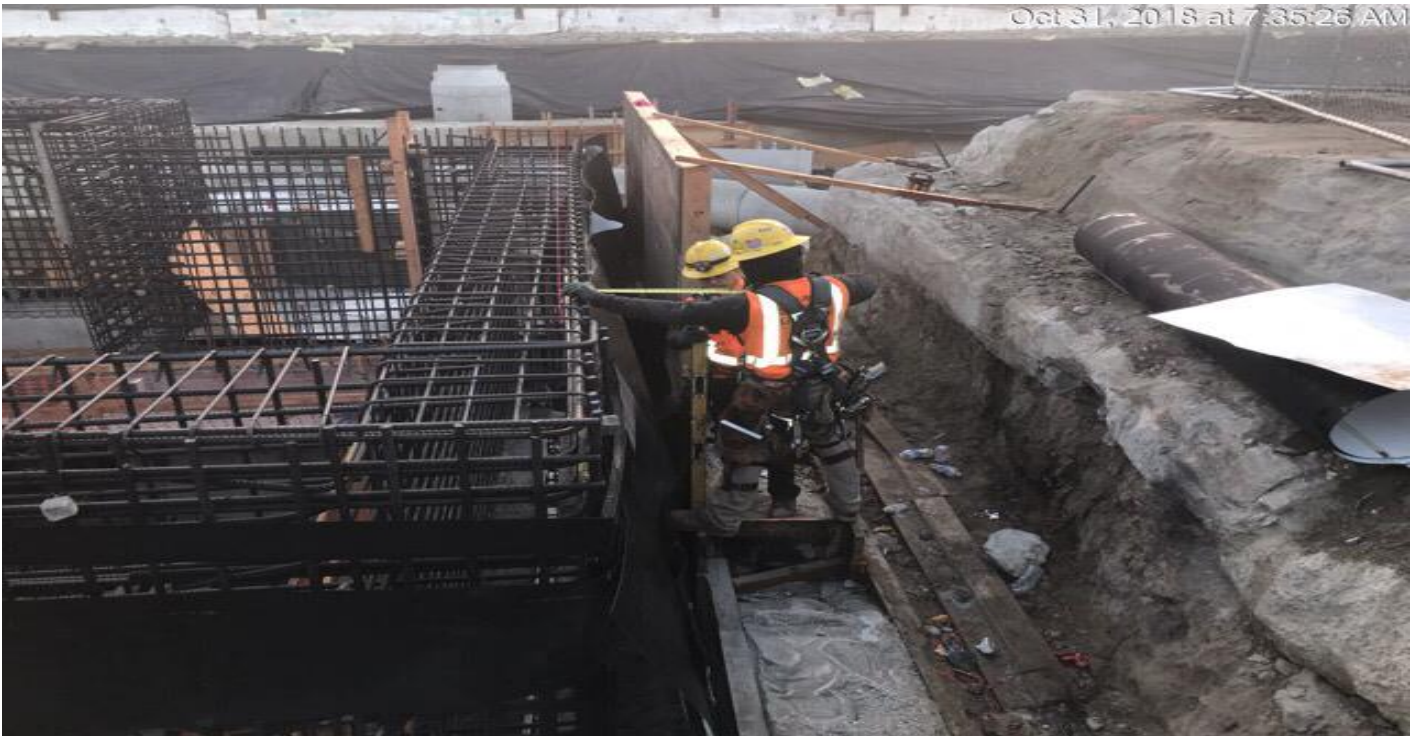
MARTIN LUTHER KING JR. STATION Installation of formwork for the walls at the elevator shaft.
