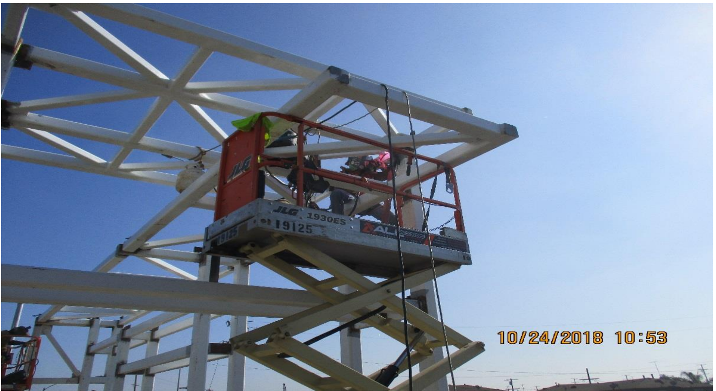
WEST STATION - Welding brackets and plates in process at the east ticket far gate at the West Station.
