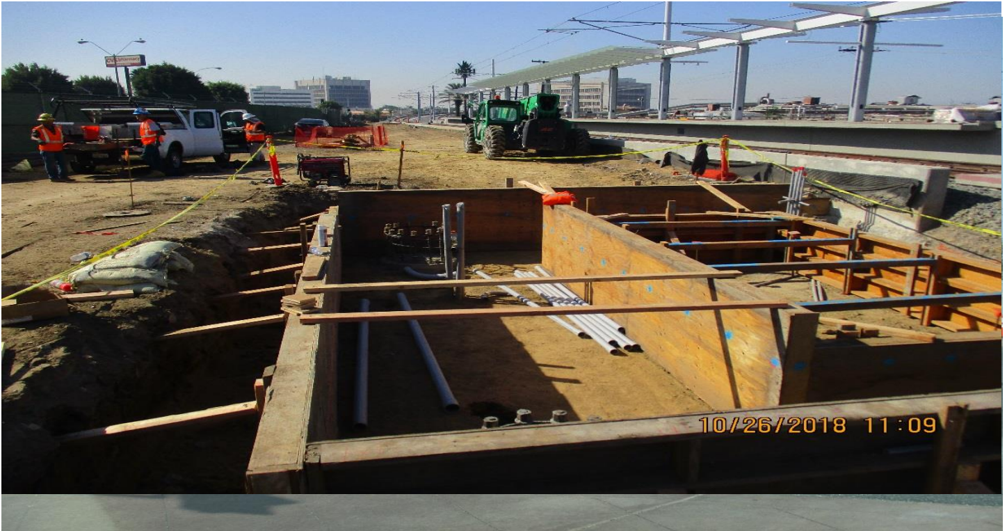
DOWNTOWN INGLEWOOD STATION - Forming completed at the Inglewood Station east fare gate.
