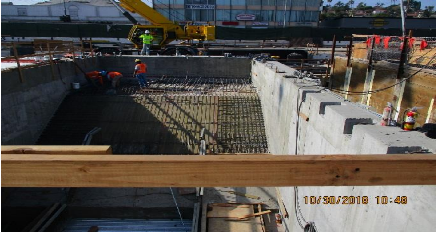
LEIMERT PARK STATION – Installation of rebar for Stairs 1 and Escalator 1 & 2 at the Entrance Structure
