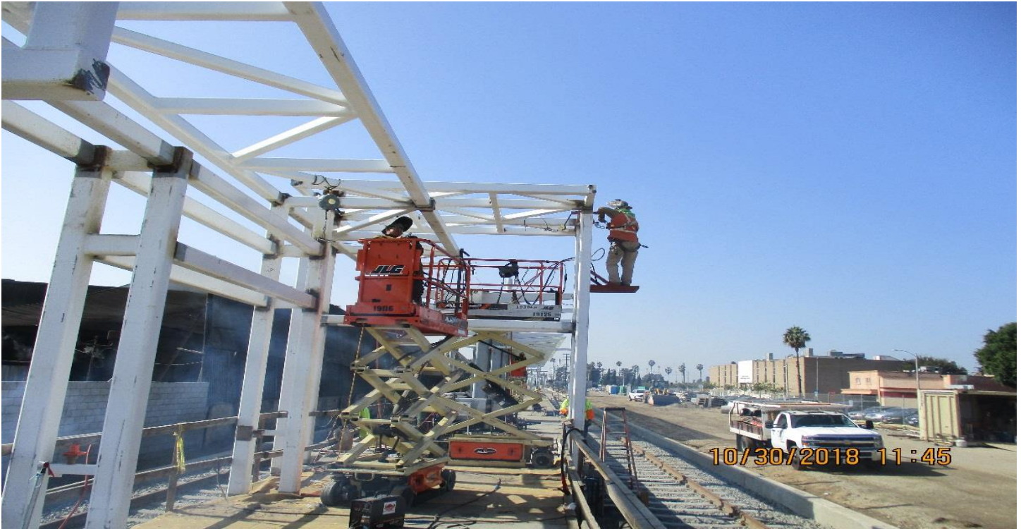
WEST STATION - Welding brackets and plates in process at the east ticket far gate at the West Station.
