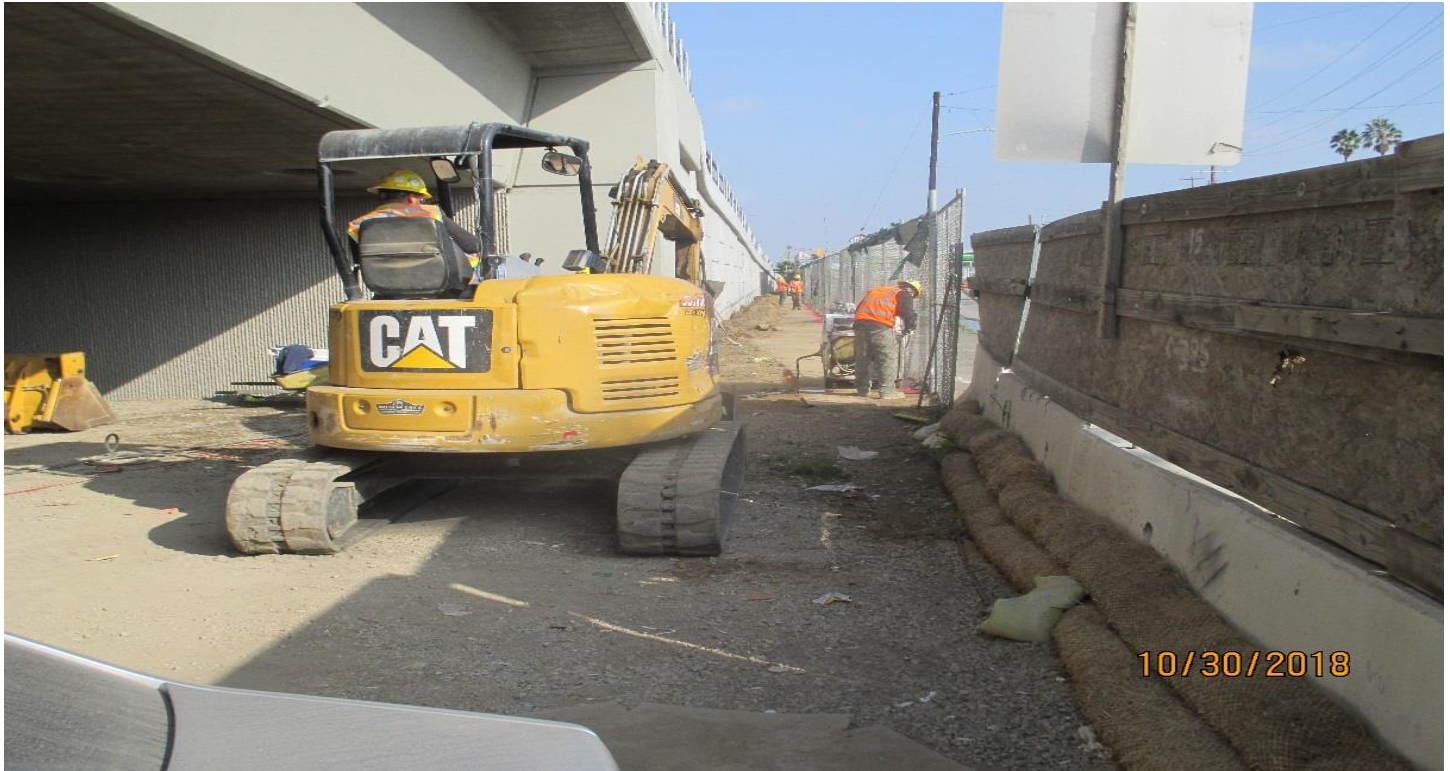
MSE 75L&R- Saw cutting the existing sidewalk to grade the NB side of RW #75.
