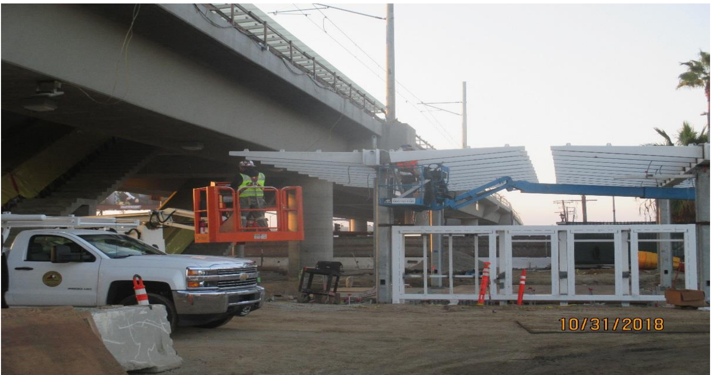
AVIATION/CENTURY STATION- Rain gutter installation for the Aviation Station ticket kiosk canopy.
