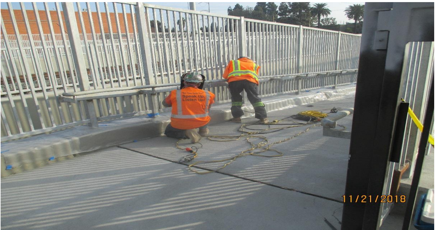
(AG-7) FCBC PED UP- Grinding the burrs from the FCBC walkway underpass hand rails.
