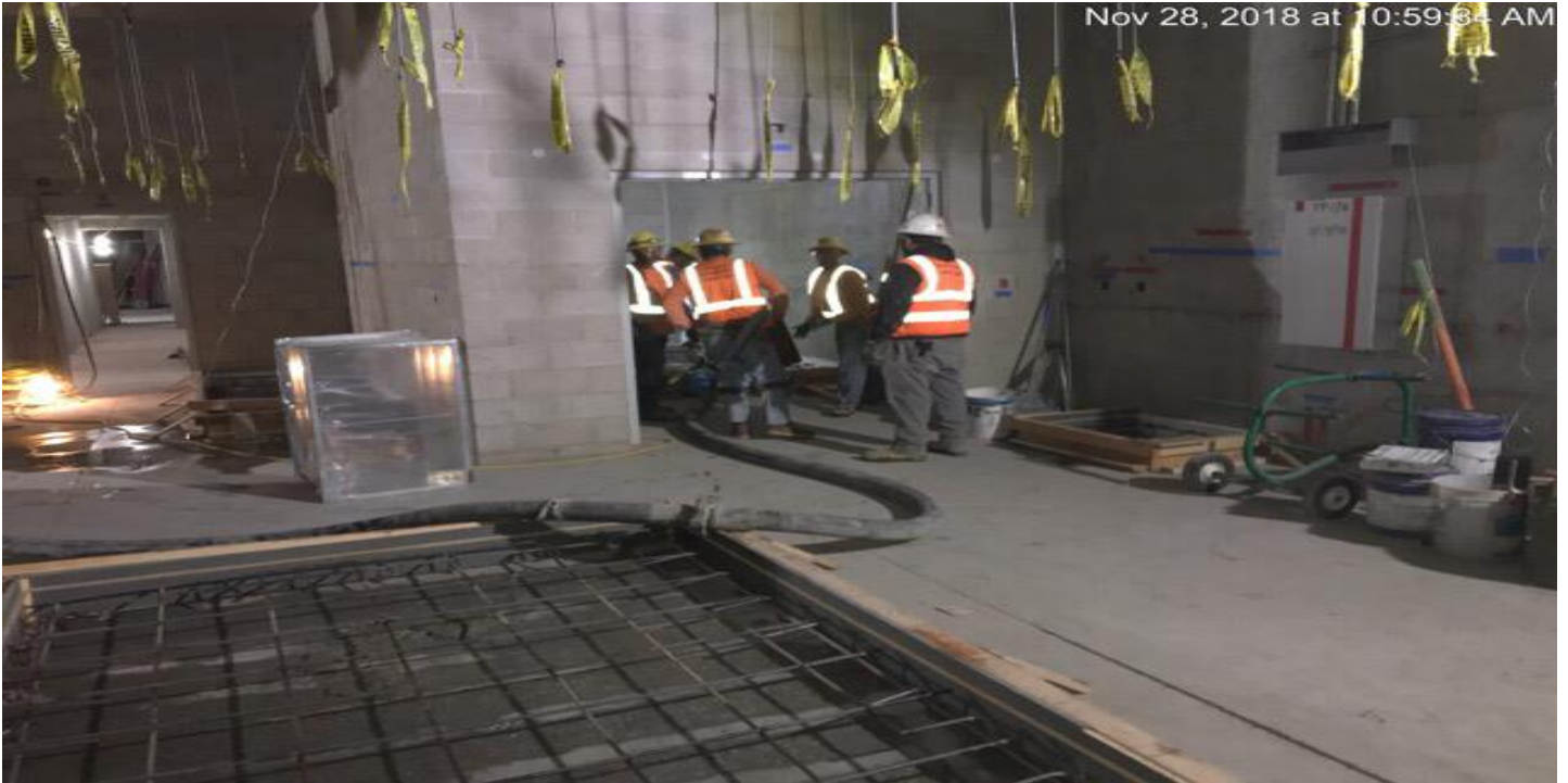
MARTIN LUTHER KING JR. STATION- Concrete placement for equipment pads in Aux Power Room North at concourse level.
