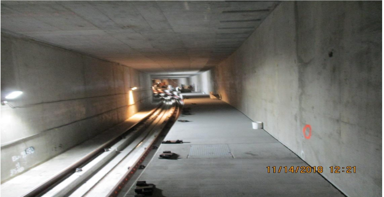
UG4 – Southbound tunnel looking north (No change since the 15th progress photos)
