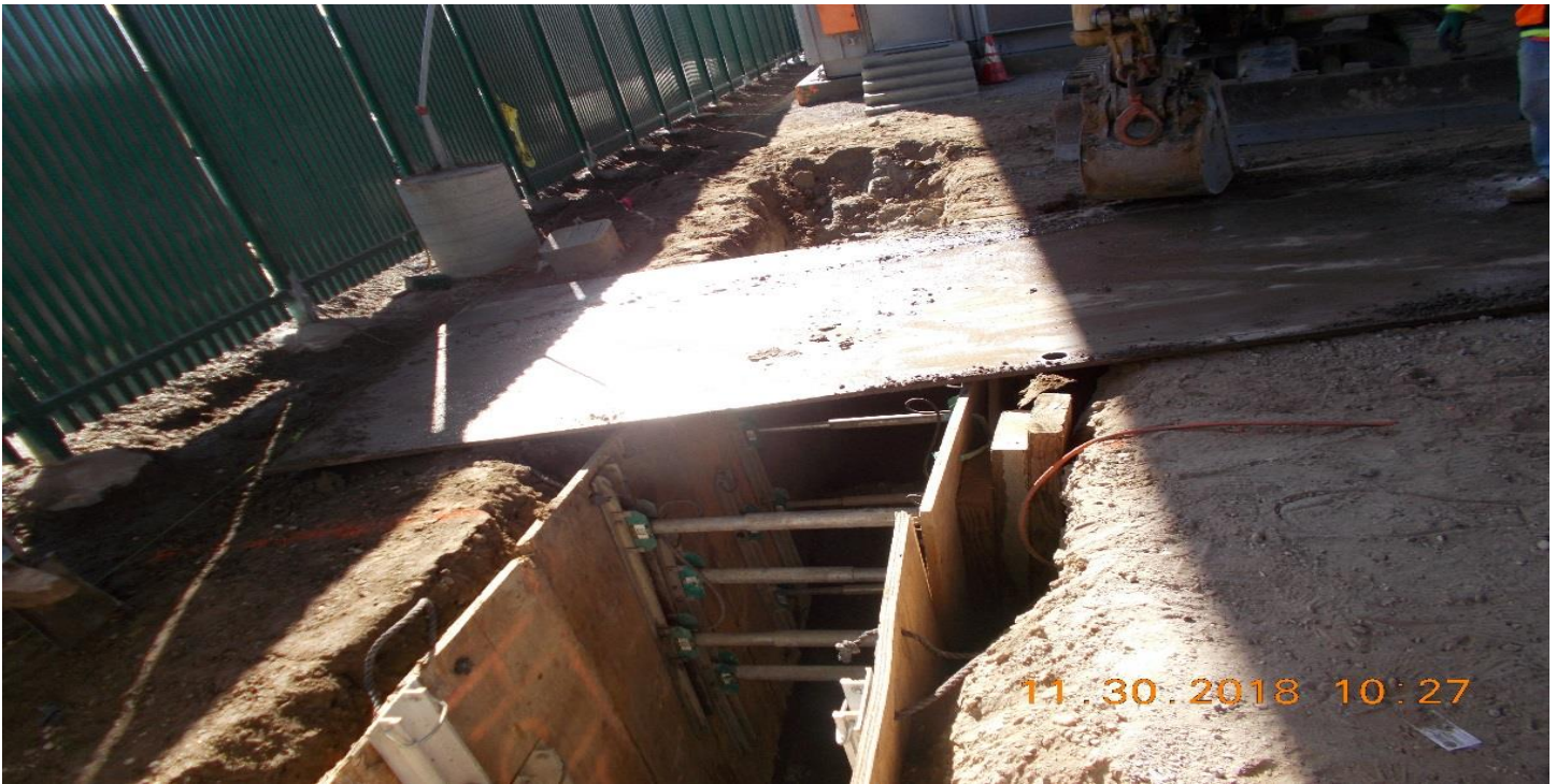
TPSS- TPSS #2. WSCC continued with excavation and added shoring to the trench.
