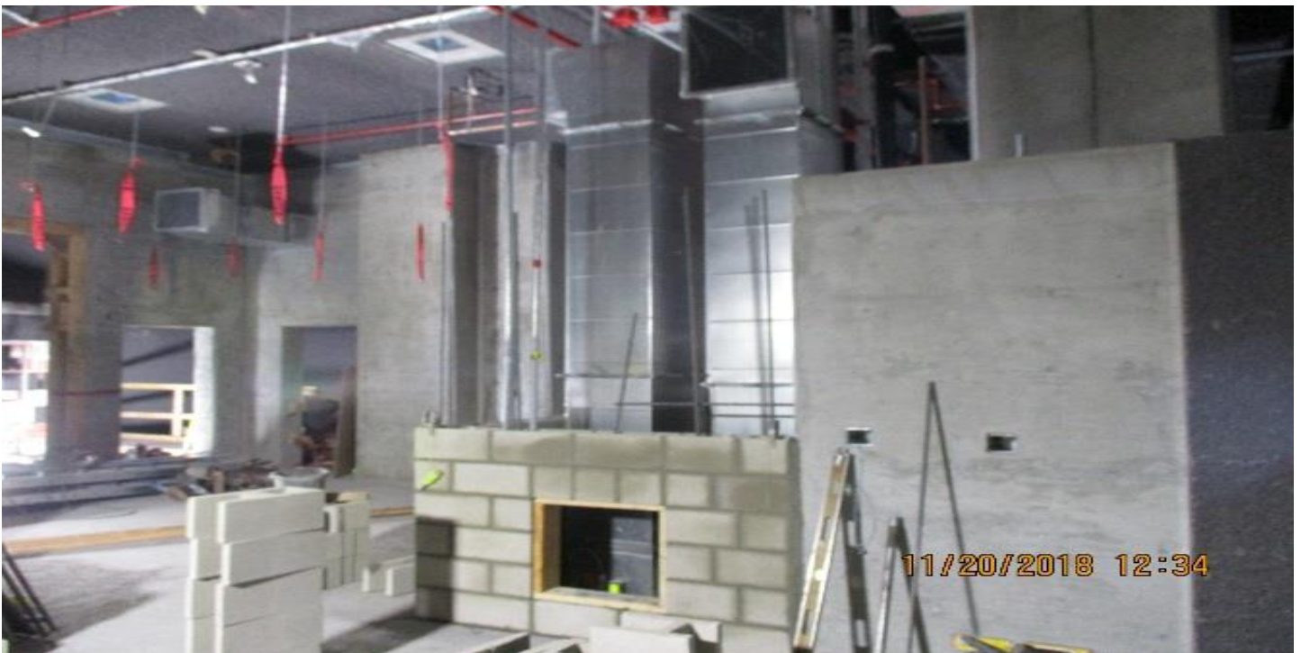
LEIMERT PARK STATION – Installation of CMU at ventilation duct niche south of Emergency stair #1 at the concourse level.
