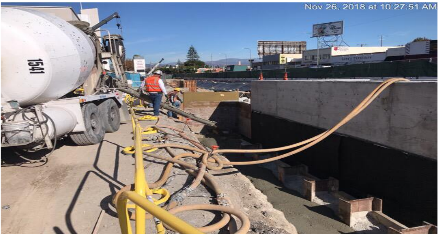
MARTIN LUTHER KING JR. STATION- Placement of slurry backfill around Emergency Vent South.
