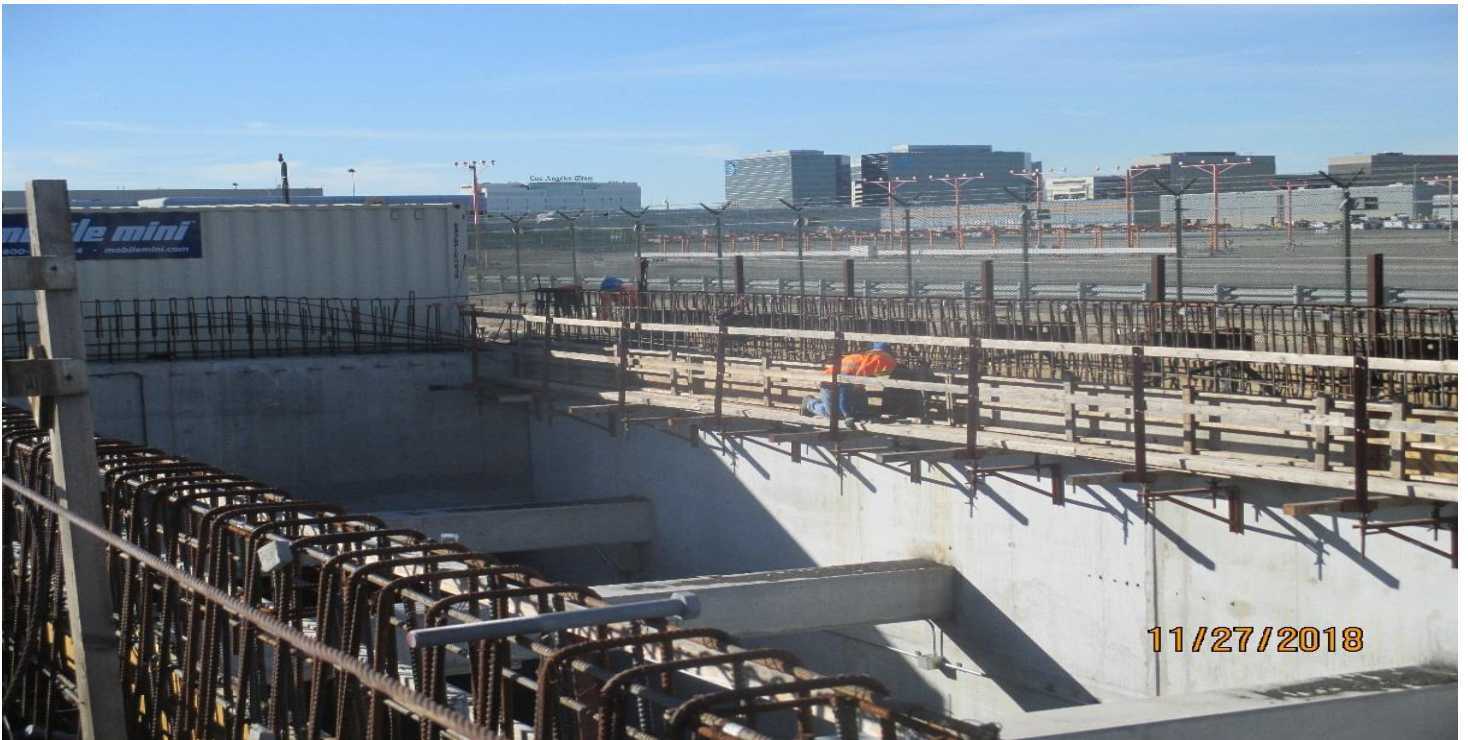
UG1- Anchor bolt installation as per RFI #2568A at UG-1 from sta. 42+00 to 45+00.
