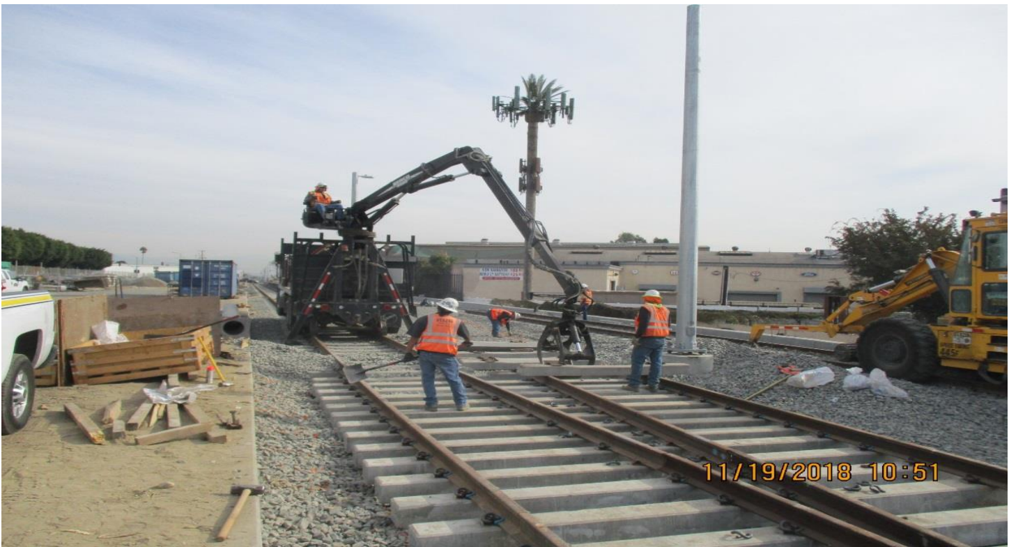
B1 GUIDEWAY - B1 Guideway between High St. and West Station placement of concrete ties for T1-T2 crossover.
