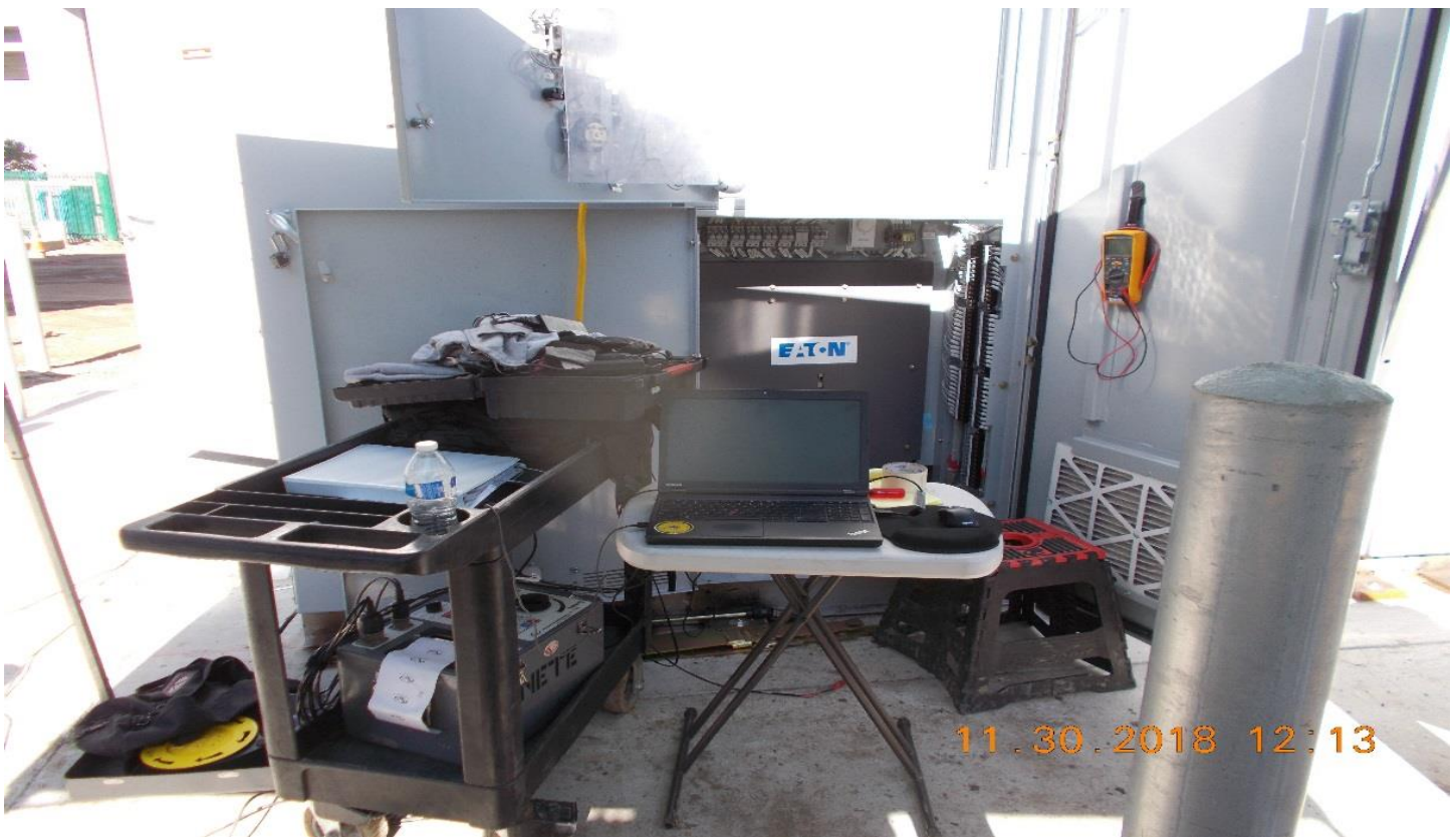
TPSS- TPSS #1. Metering gear Field Acceptance Test (FAT) testing by N.E.T.E
