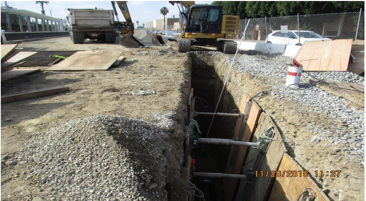
FAIRVIEW HEIGHTS STATION - Excavating and laying 12" sub drain line at the Fairview Station.
