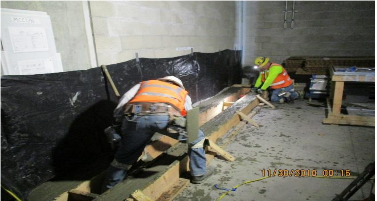
LEIMERT PARK STATION – Concrete placement of equipment pads at Aux Power Room North.
