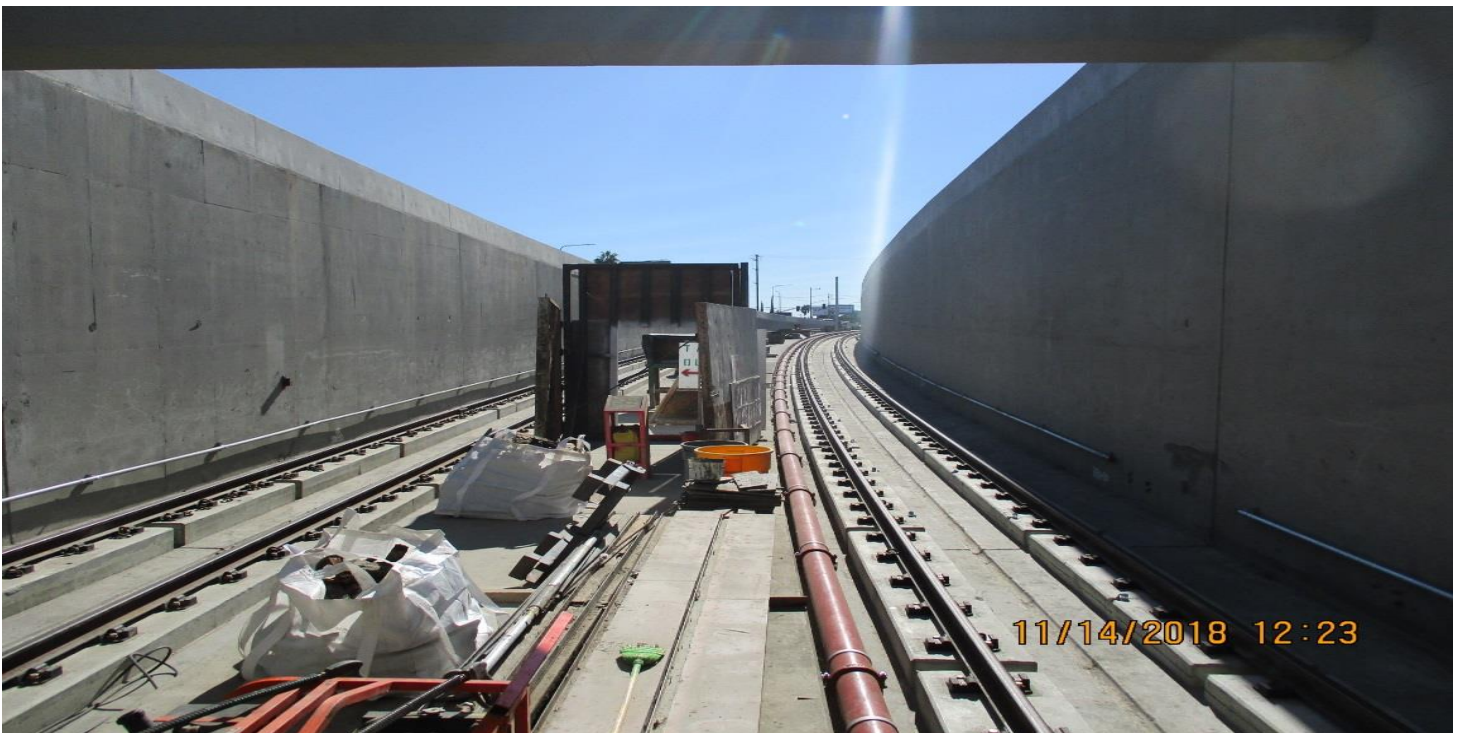
UG4 -- Tracks at the south portal looking south (No change since the 15th progress photos)
