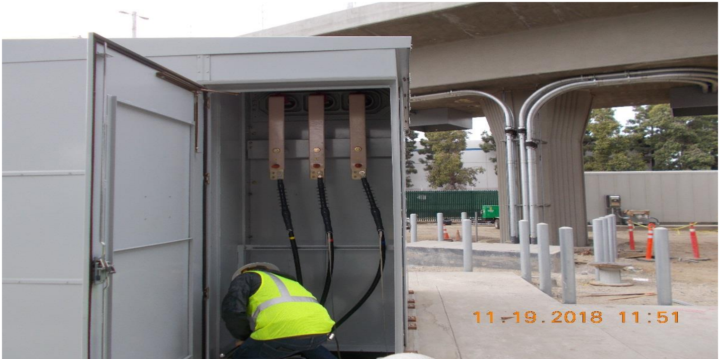
TPSS- TPSS #1. Cables from metering gear to A01 have been hi-potted, terminated, & now being landed.
