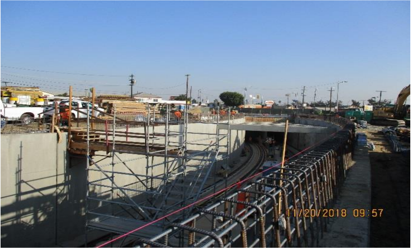
UG3 - Installation of rebar for the barrier wall on the above the U-channel walls between P2 and P-11.
