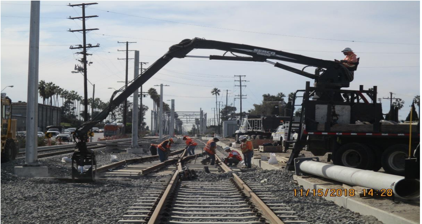
B1 GUIDEWAY - B1 Guideway at High St. to West Sta. T1 crossover.
