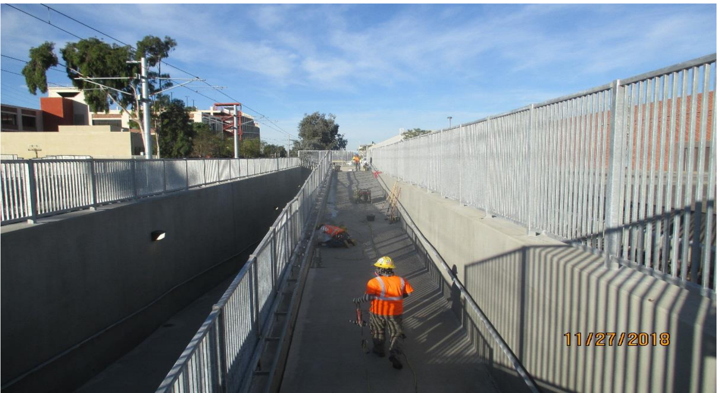
(AG-7) FCBC PED UP- Finish concrete and steel hand rail work for the SB side of the FCBC.
