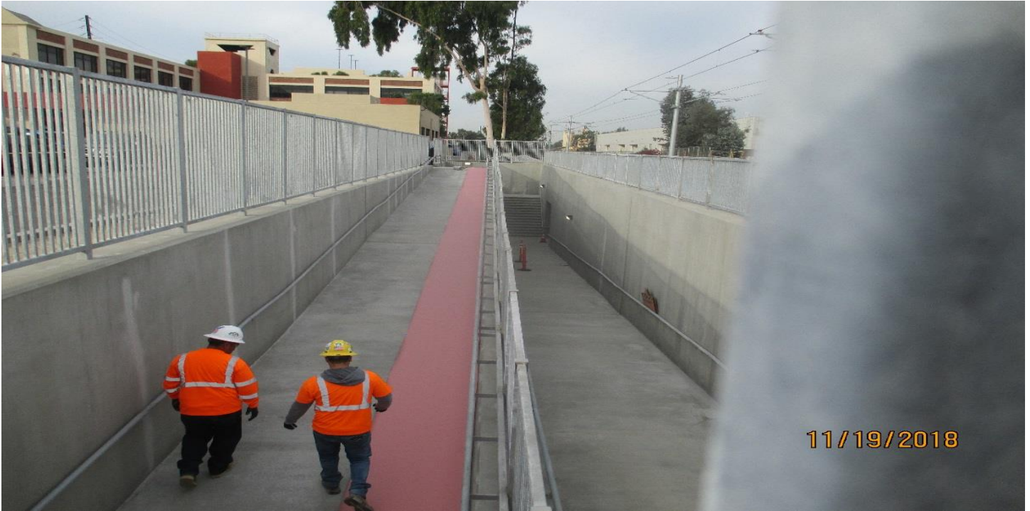
(AG-7) FCBC PED UP- Prepping to fog the concrete finish of the NB side of the FCBC walkway.
