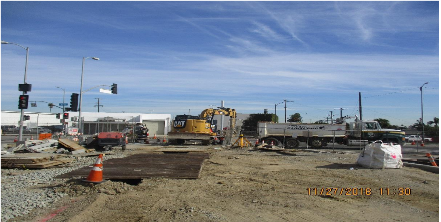
FAIRVIEW HEIGHTS STATION - Excavating for a new catch basin at the Fairview Station.
