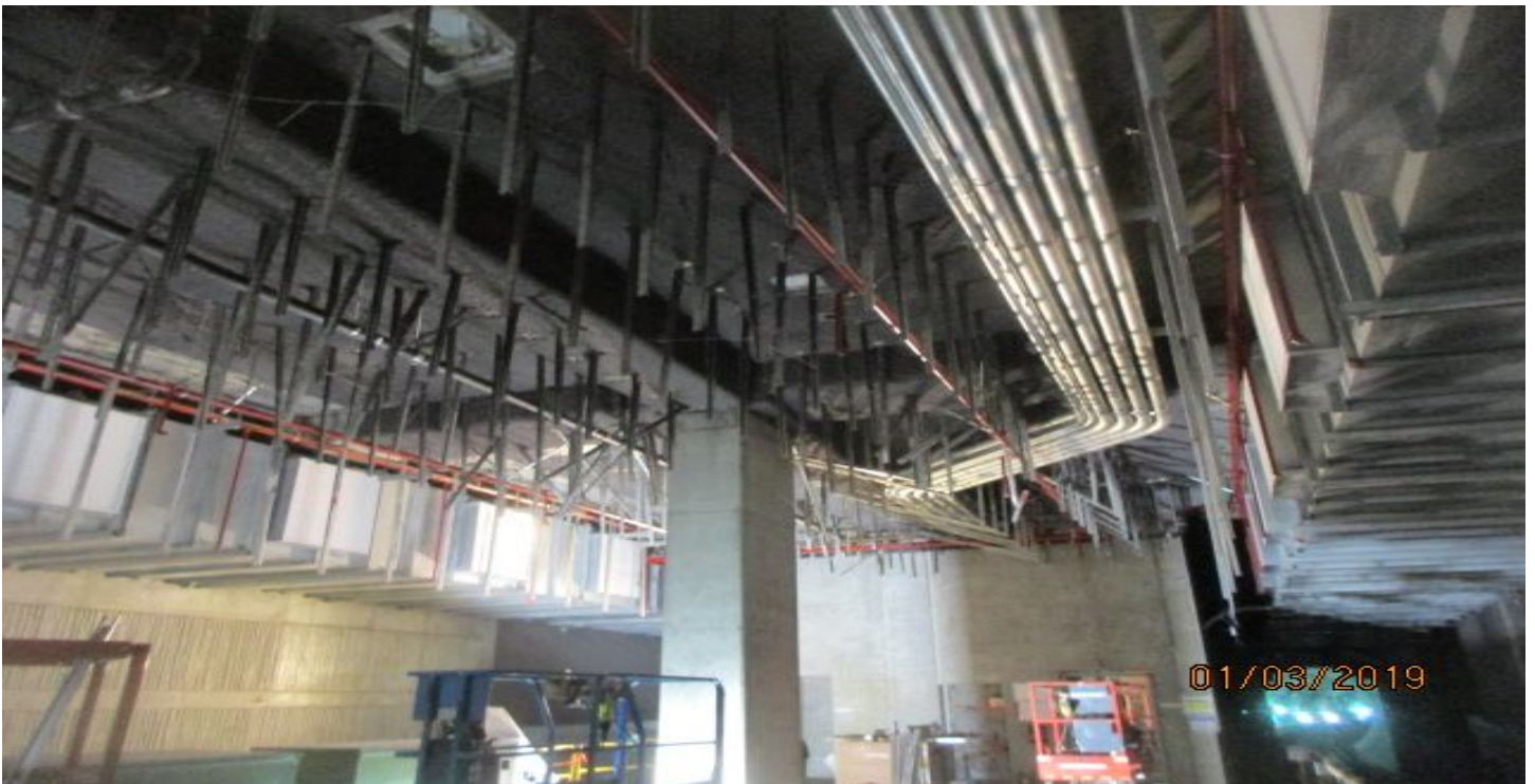
LEIMERT PARK STATION – Metal ceiling hangers for the ceiling above the platform.
