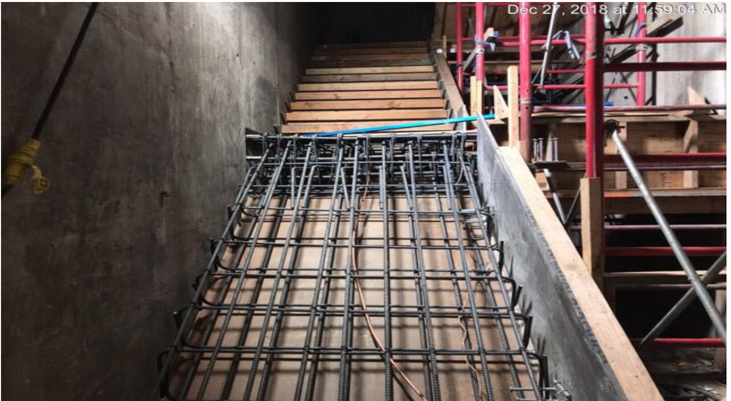
EXPOSITION/CRENSHAW STATION – Installed of rebar and formwork for Emergency Exit Stairs #2 North.
