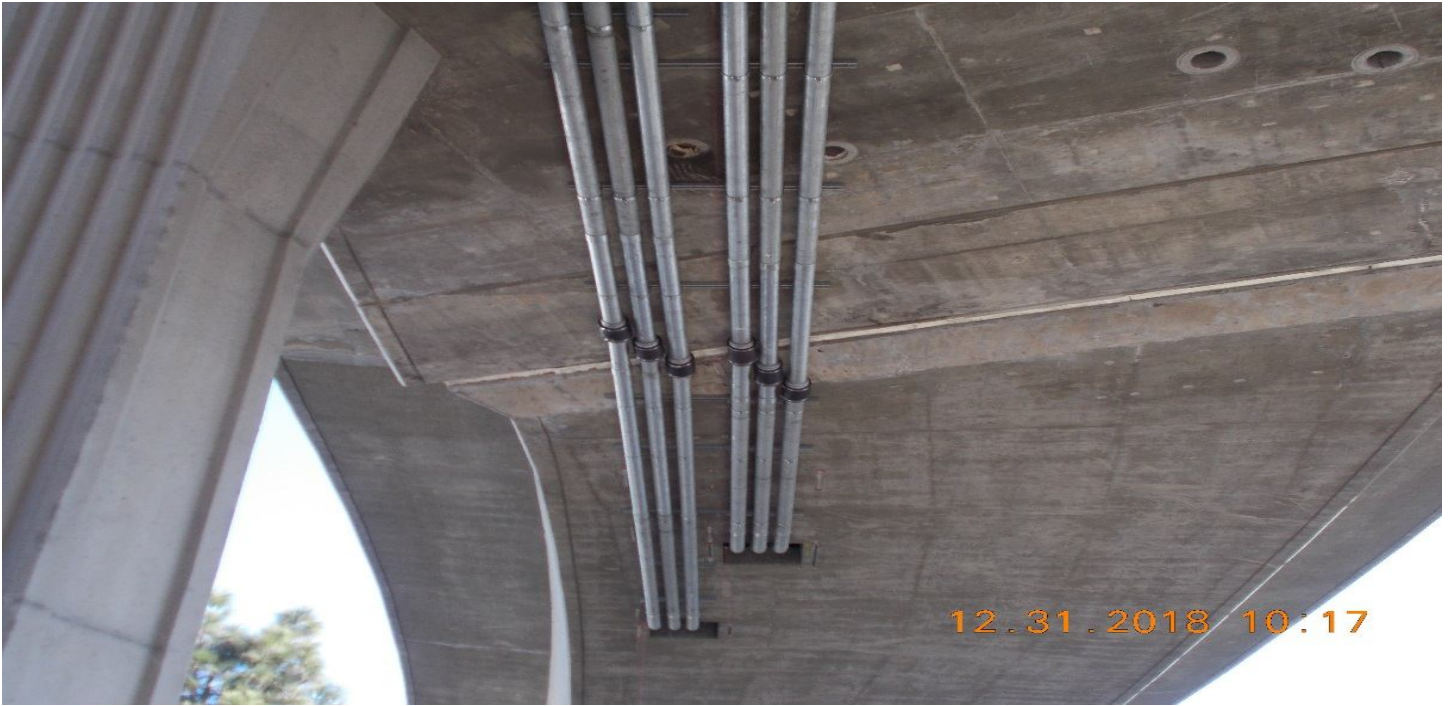
TPSS- TPSS #1. Traction 4-inch conduits with kink in expansion couplings.
