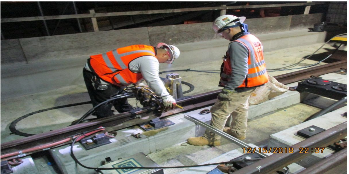
GREENLINE UNDERPASS- BJ install, layout of restraining rail, and coring for skewed fasteners at Hinge 14.
