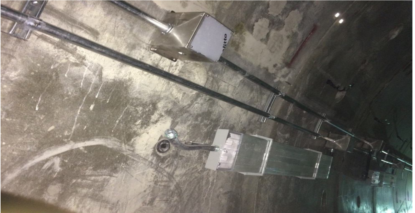
TUNNEL – Emergency lighting in the northbound tunnel between Expo and MLK Station.
