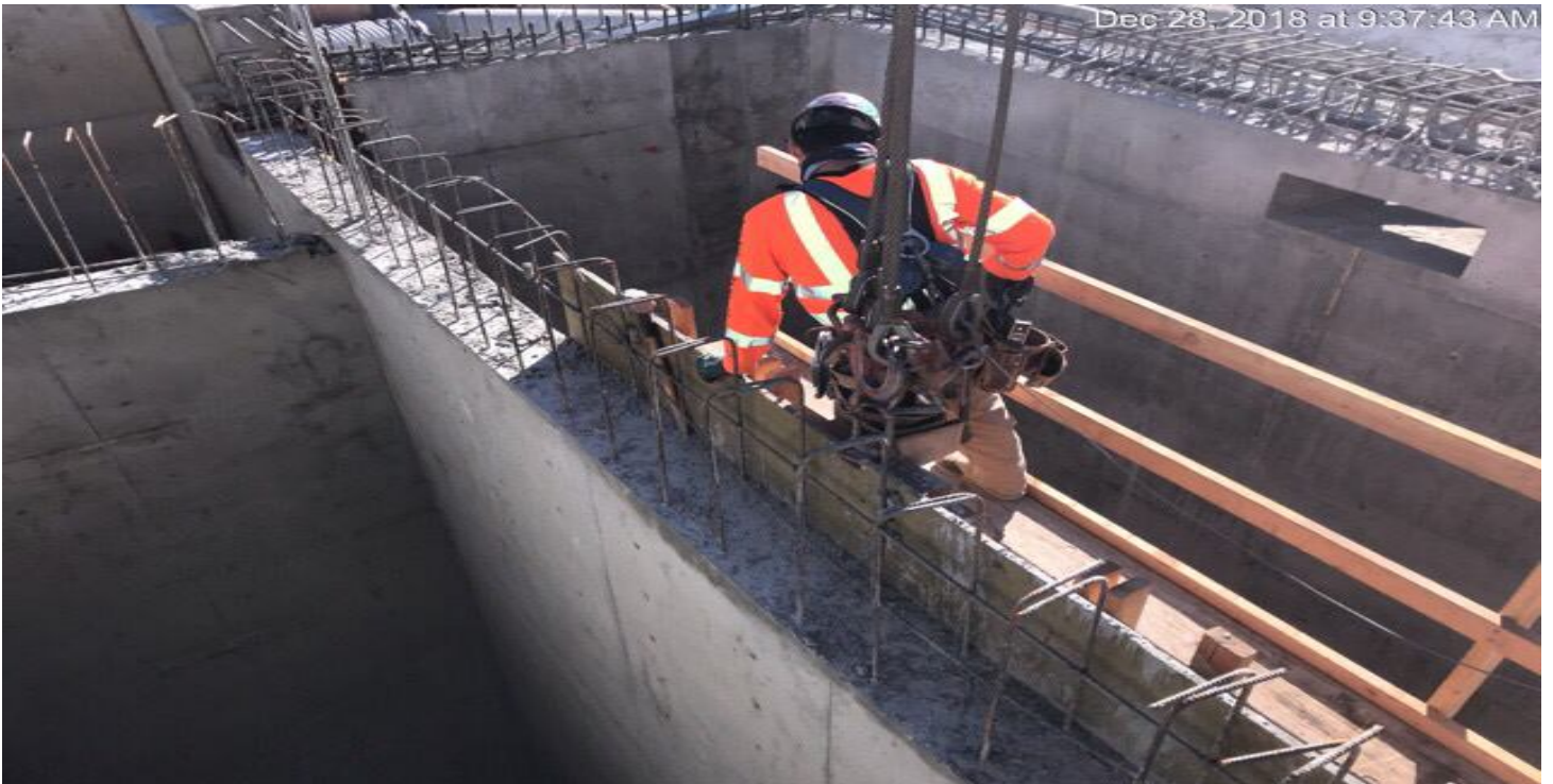
MARTIN LUTHER KING JR. STATION- Removal of formwork from the interior elevator walls at the roof level.
