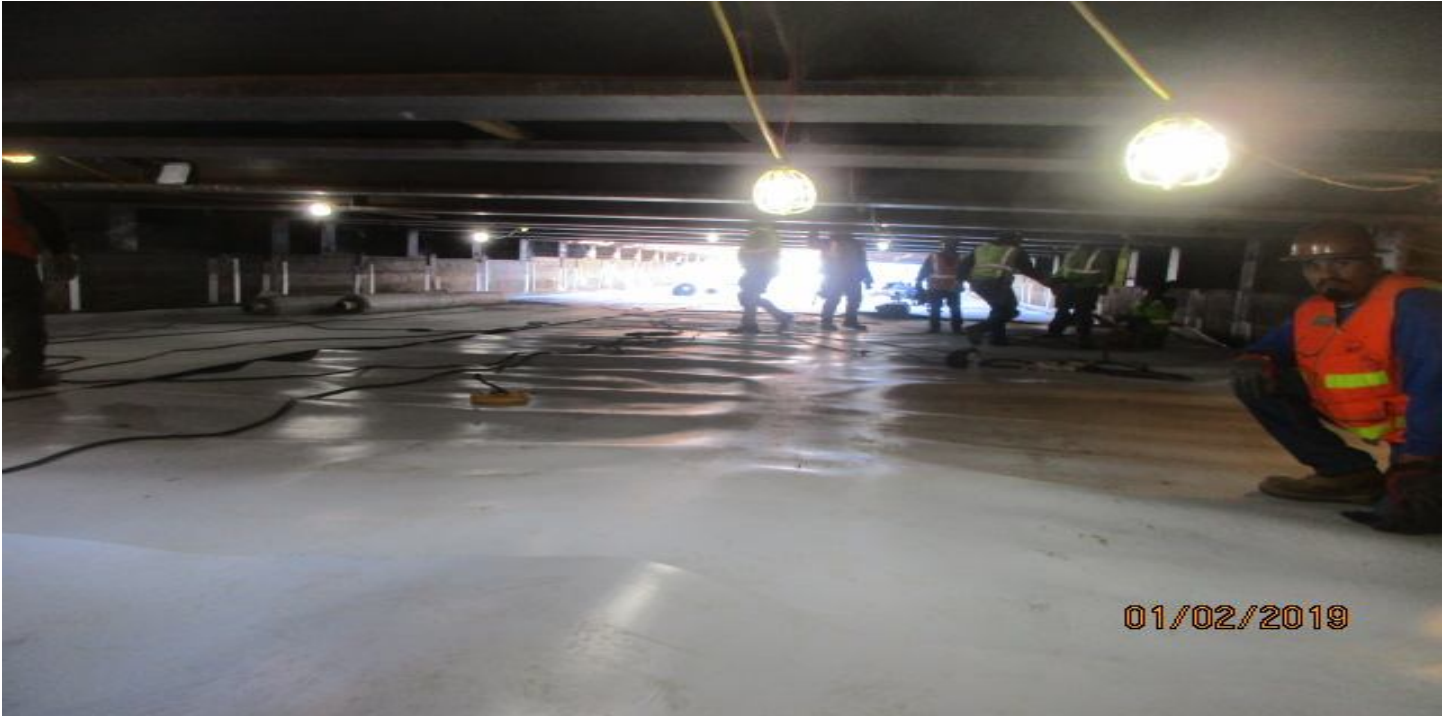
UG3 - Waterproofing above the roof underneath the deck panels at 67th street.
