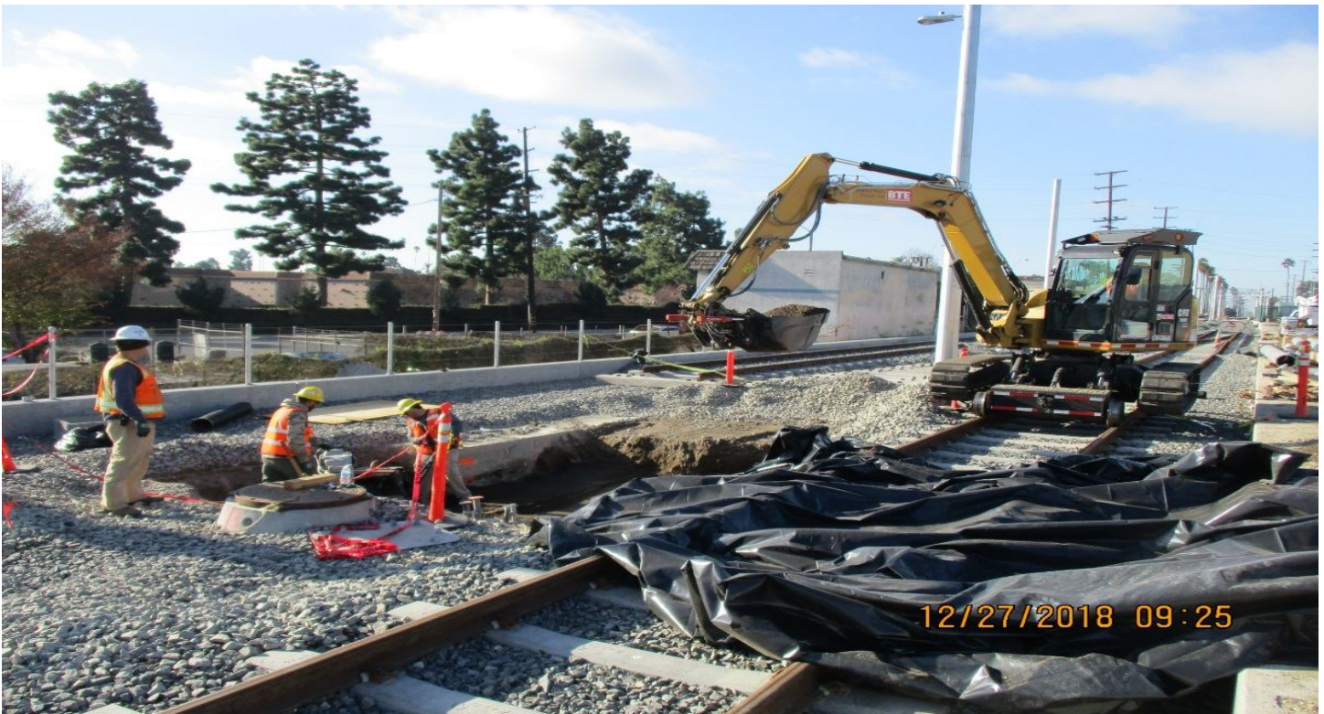
B1 GUIDEWAY - B1 Guideway east of West Sta backfill for pullbox relocation at T1-T2.
