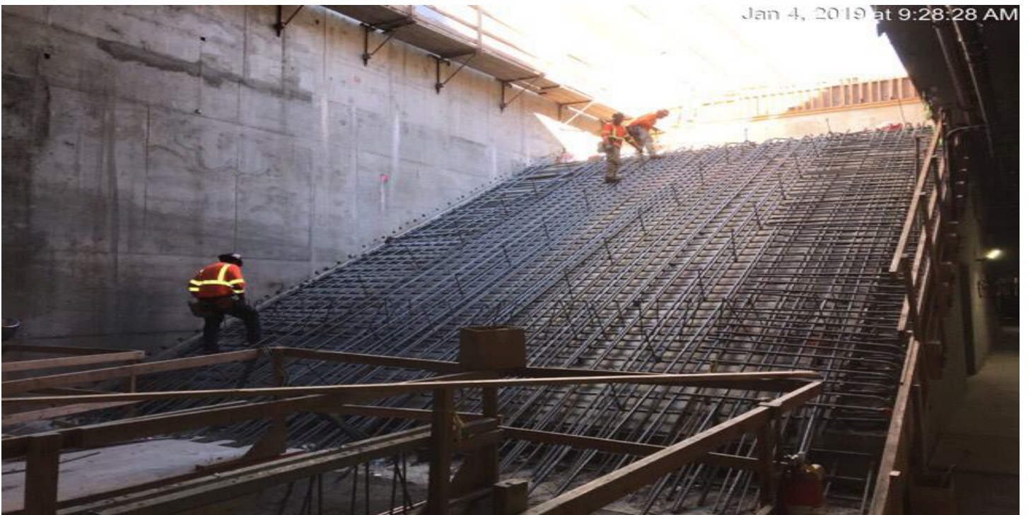
MARTIN LUTHER KING JR. STATION- Placement of slurry backfill around Emergency Vent South.
