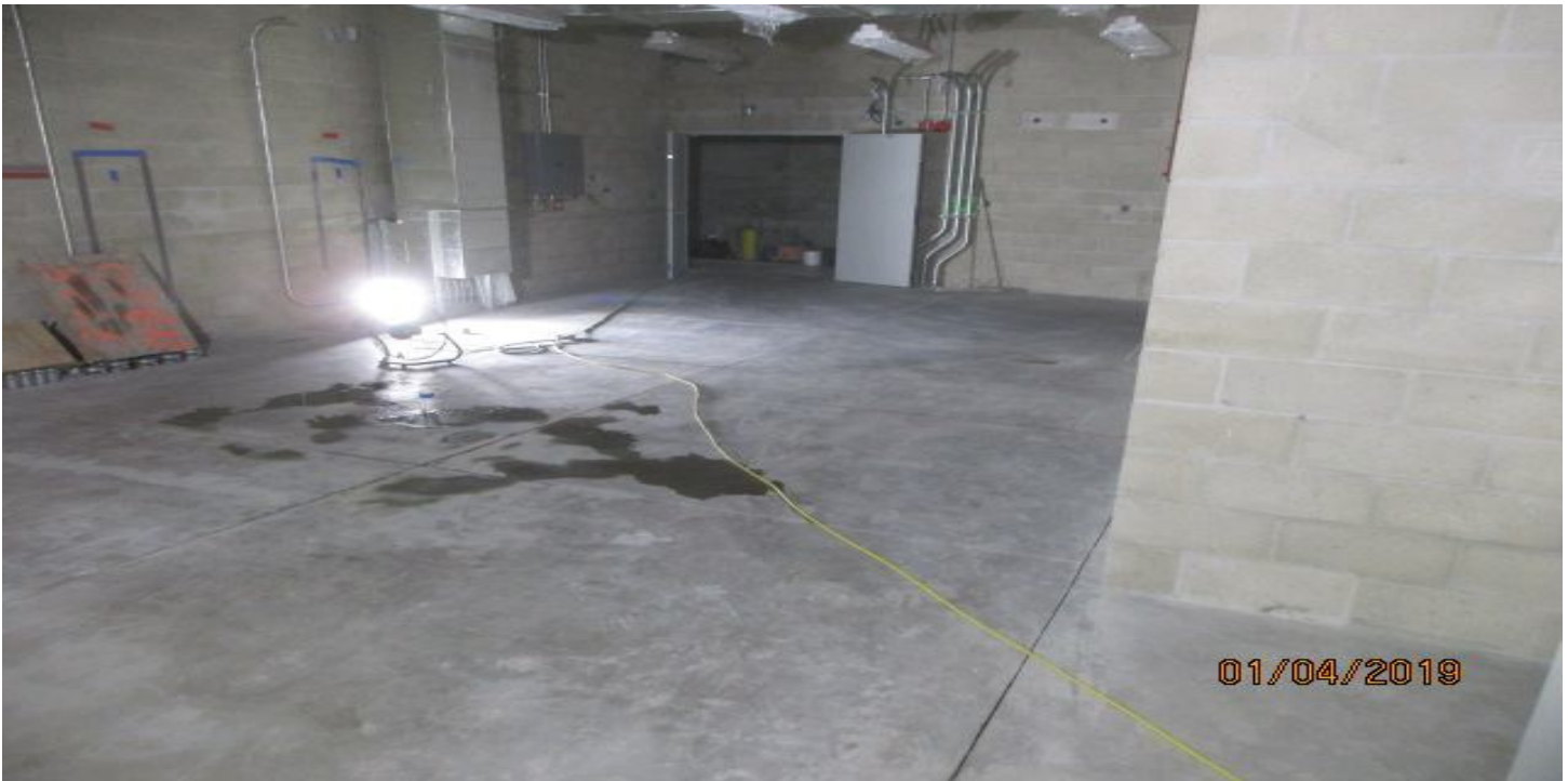
LEIMERT PARK STATION – Preparation of the floor for sealant at the concourse level TC&C room .
