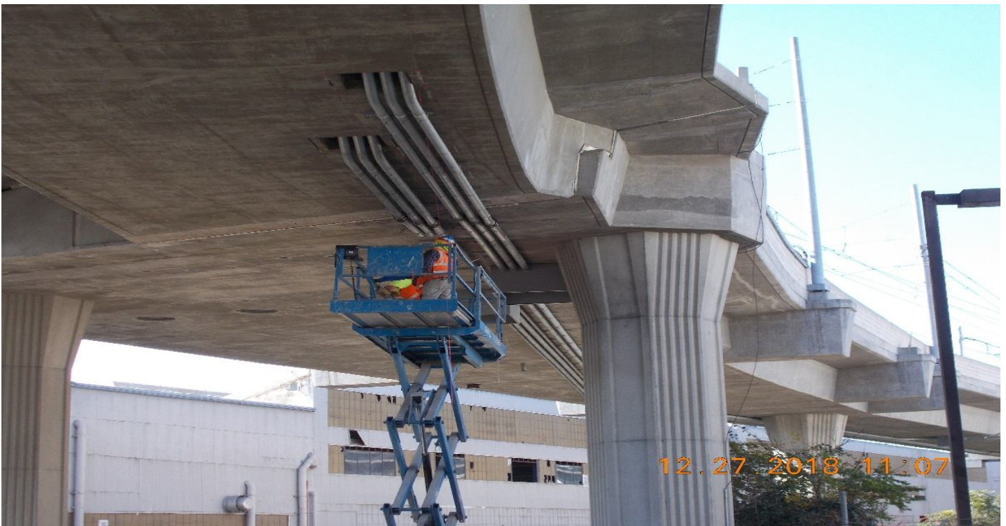
TPSS- TPSS #1. WSCC Electrical continues to run traction 4-inch across Hornet Way.
