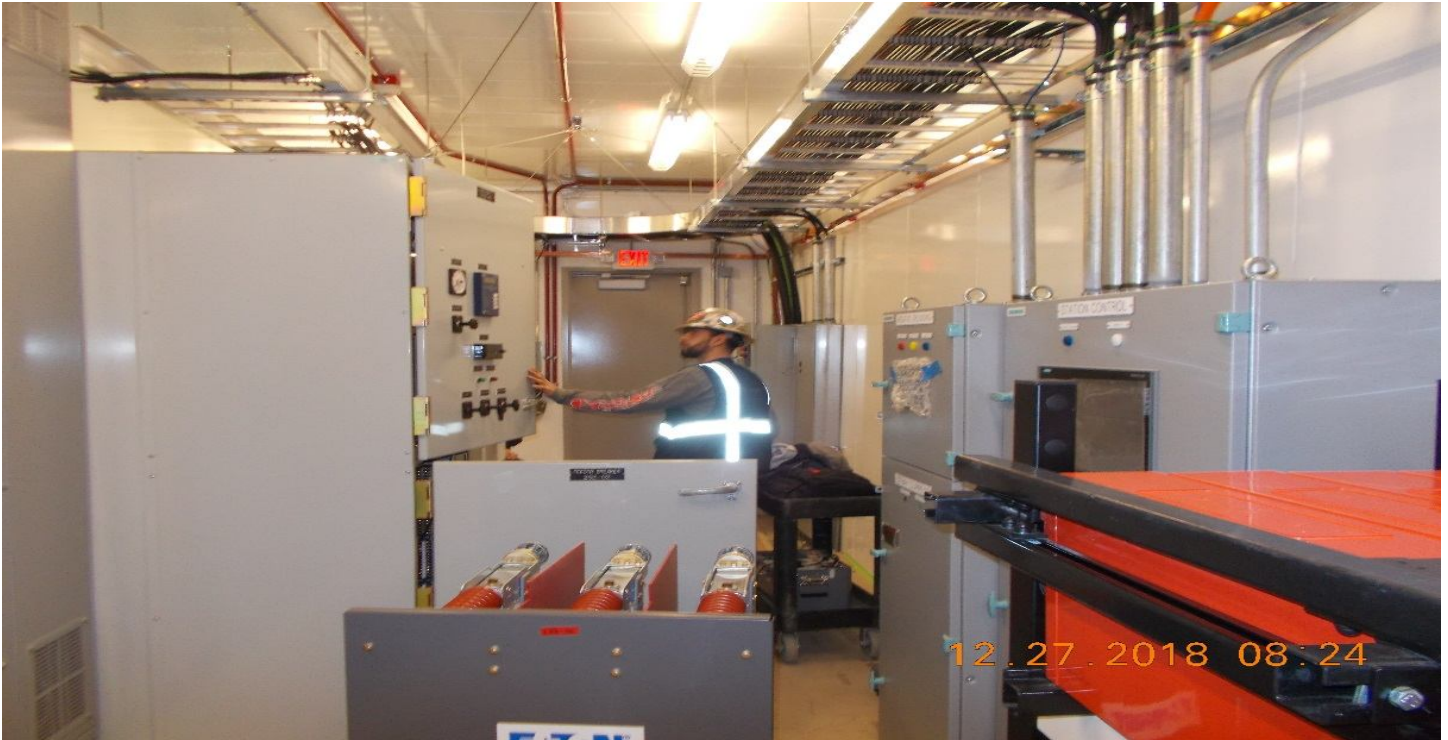
TPSS- TPSS #3. NETE was finishing AC switchgear function testing.
