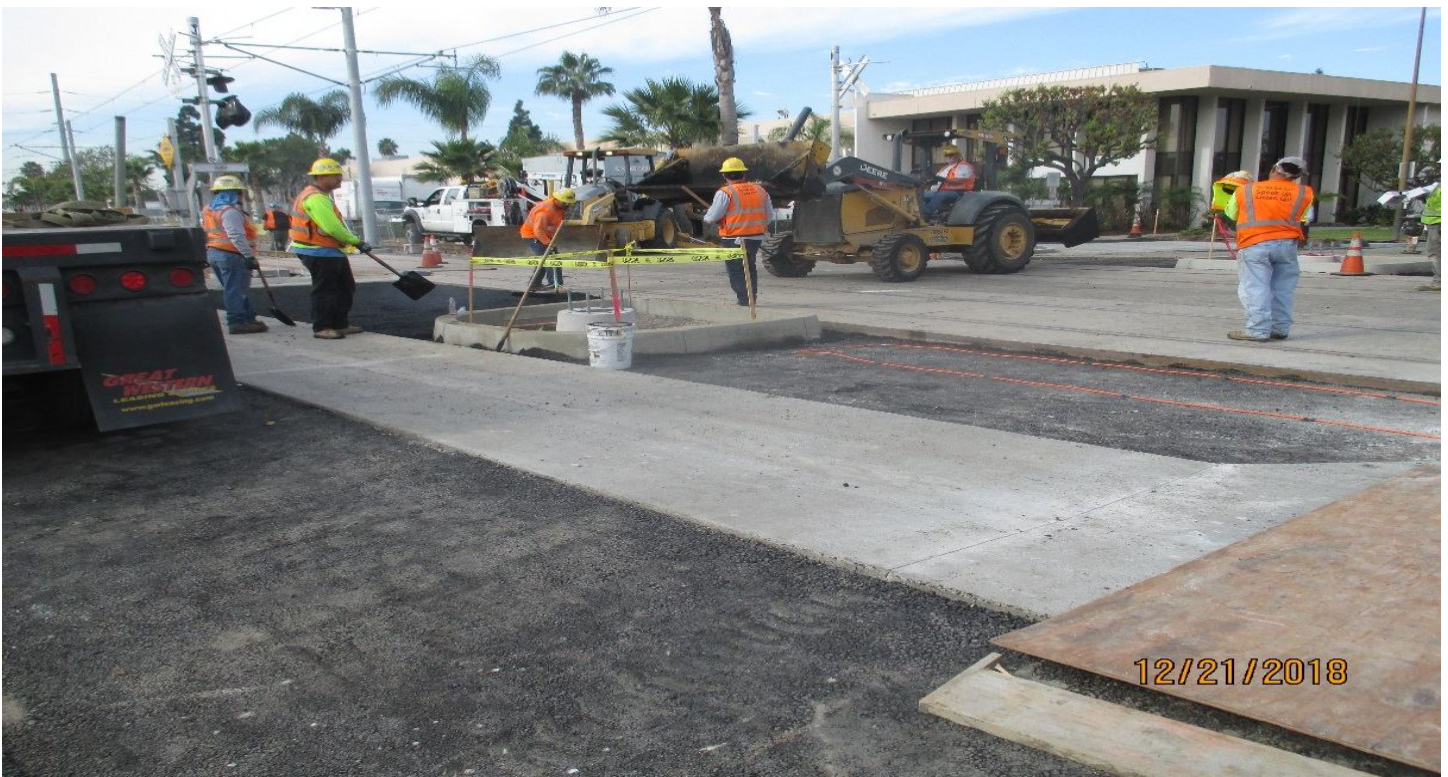
B1 GUIDEWAY - VDL loops placed and AC being placed over them on Oak.
