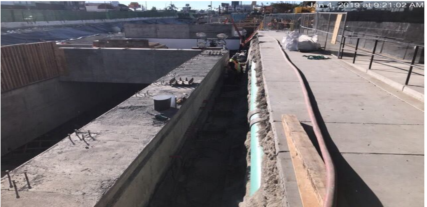
MARTIN LUTHER KING JR. STATION Installation of waterproofing for the west plaza wall.
