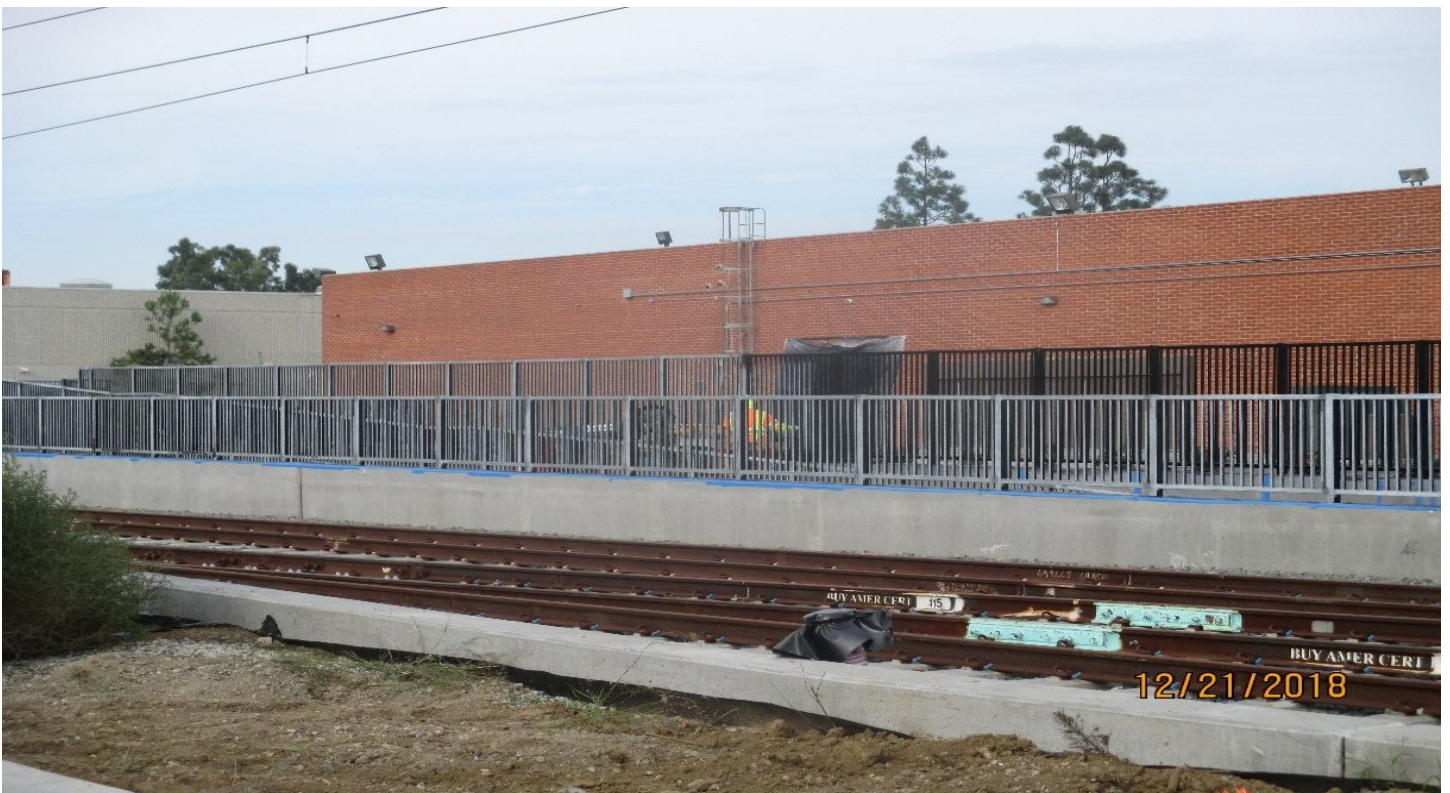
(AG-7) FCBC PED UP- Applying primer to the SB side of the FCBC walkway underpass.
