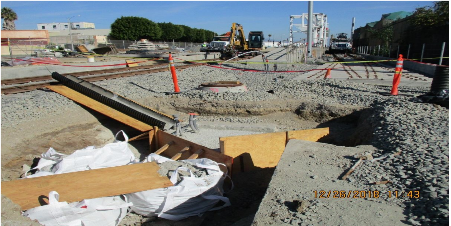
B1 GUIDEWAY - Applying primer to the SB side of the FCBC walkway underpass
