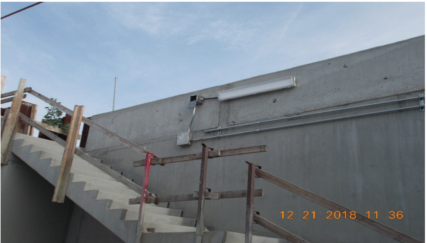
UG1- Plastic based fixtures installed at 56+50.
