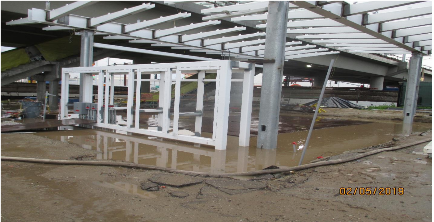
AVIATION/CENTURY- Flooding at the Aviation Station.
