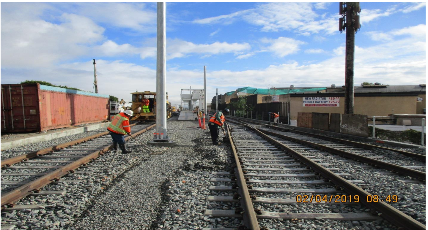
B1 GUIDEWAY - B1 guideway between High street and West blvd. surface, line, tamp, correct skewed ties and dressing ballast rock.
