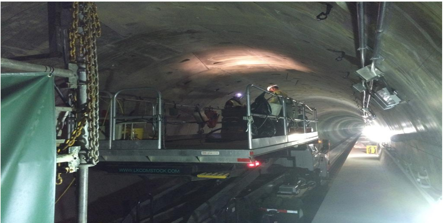
TUNNEL – Installation of support anchors in the NB tunnel between EXPO and MLK Station.
