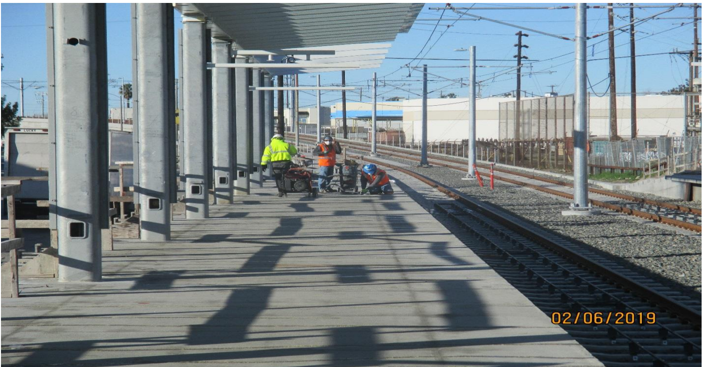
WESTCHESTER STATION- Grinding the crack seal epoxy on the NB Westchester platform deck.
