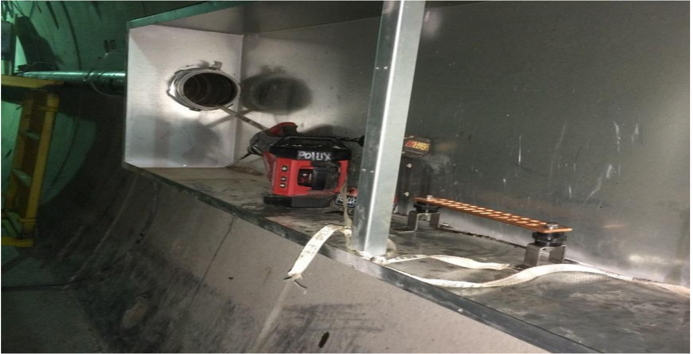
TUNNEL – Installation of electrical components at the SB tunnel between EXPO and MLK Station.
