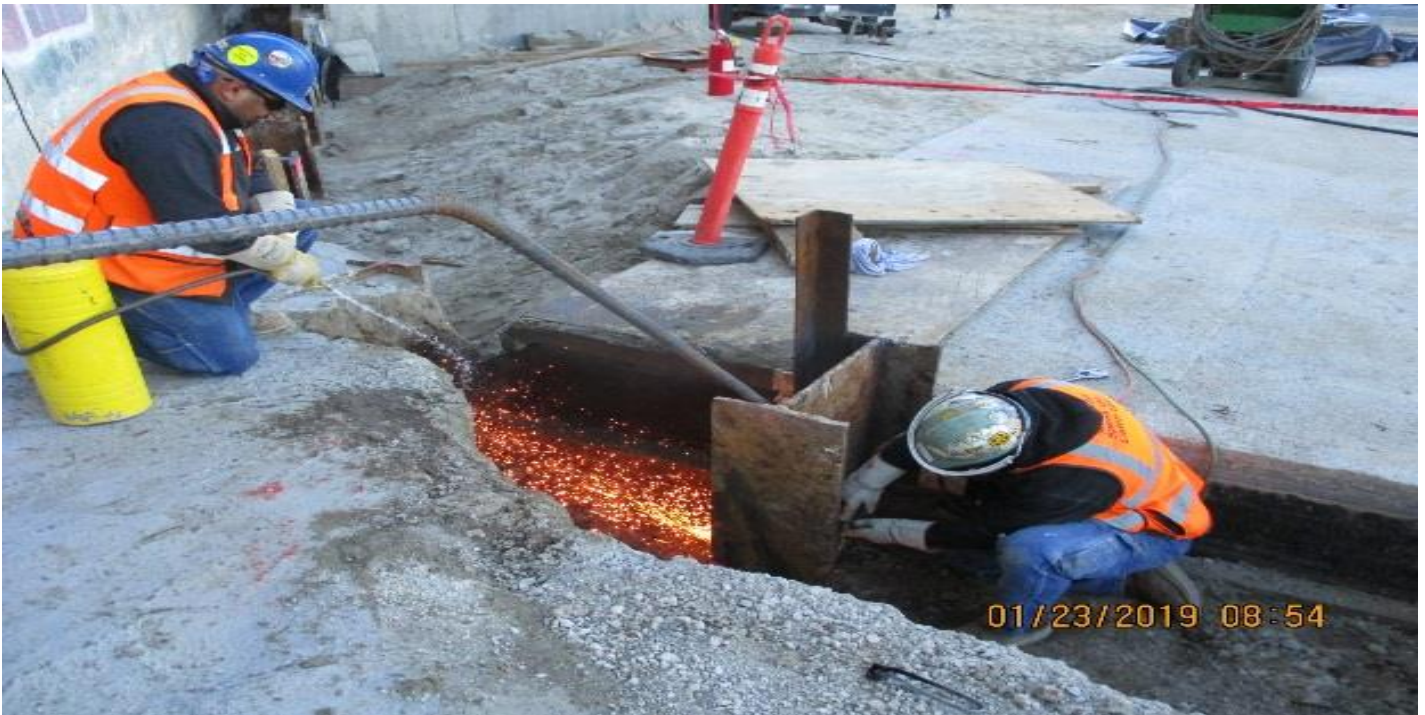
LEIMERT PARK STATION – Removal of piles along the southeast station for screen wall.
