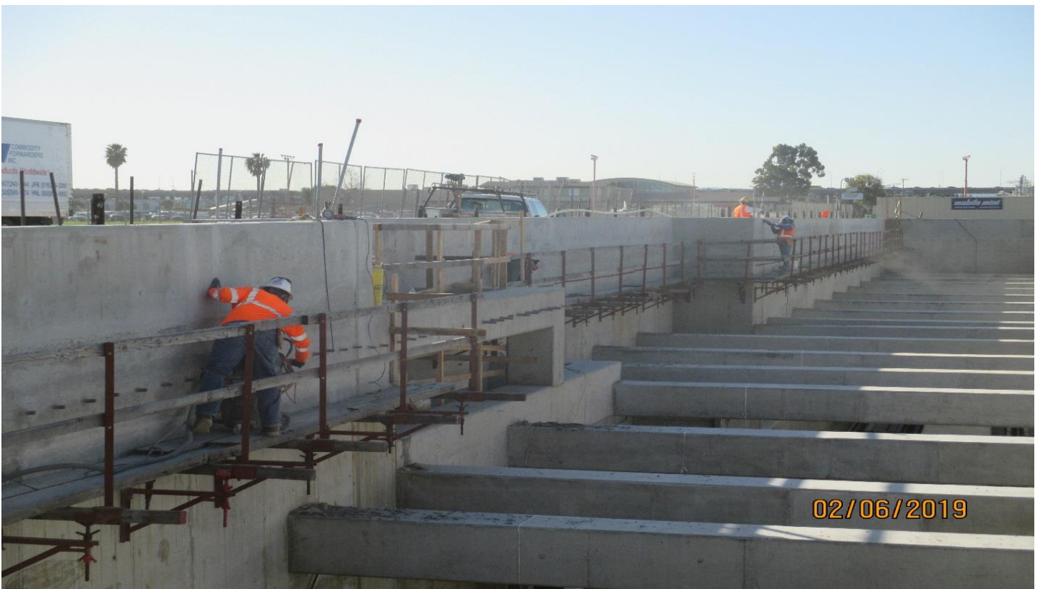
UG1- Plastic based fixtures installed at 56+50.
