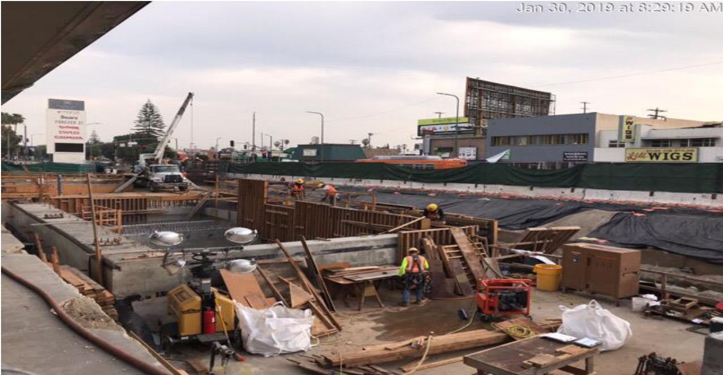
MARTIN LUTHER KING JR. STATION- Installed formwork for walls at the Plaza level.
