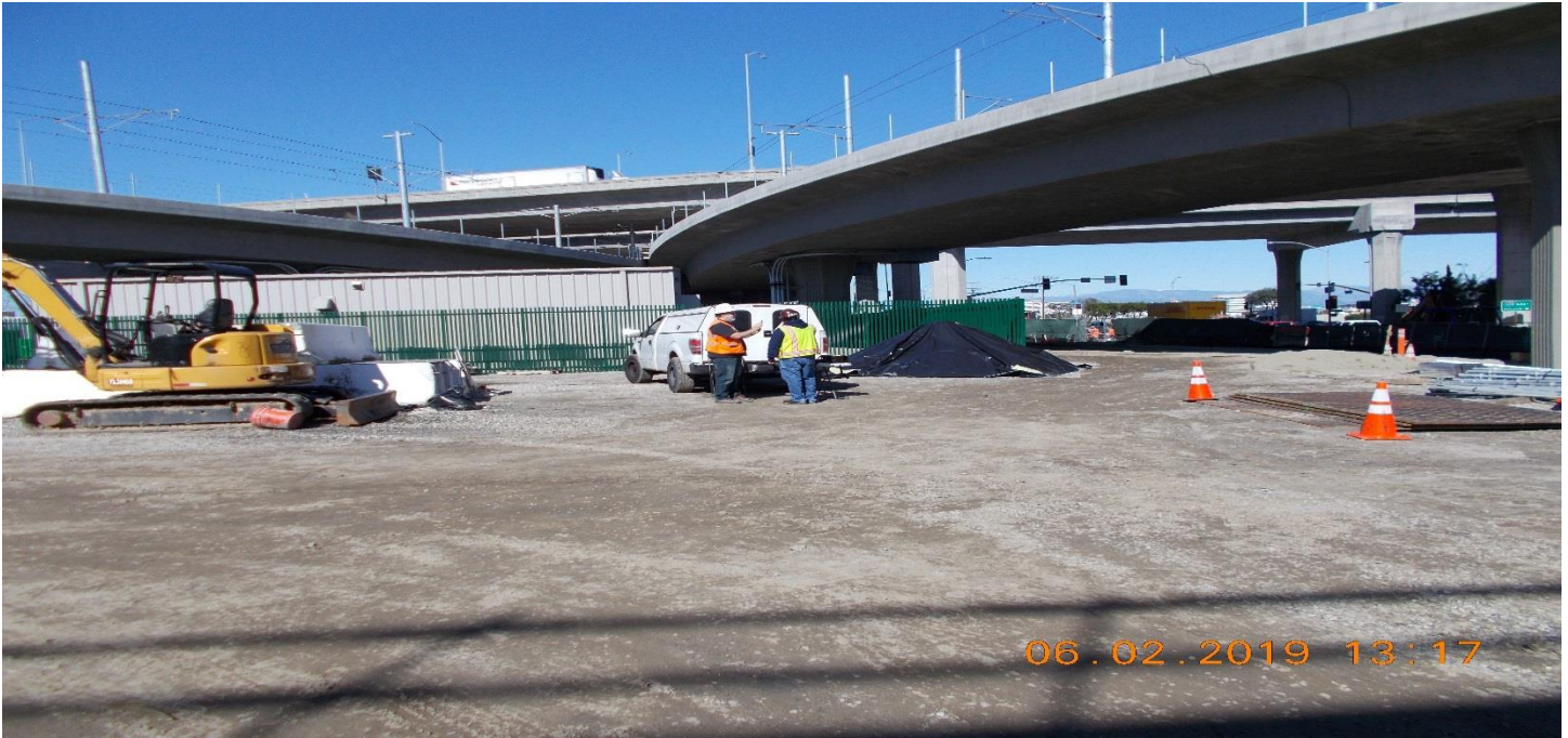
TPSS TPSS #1. NETE was re-doing the ground grid test without the TPSS enclosure grounds connected.
