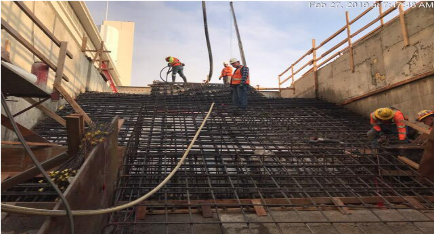
MARTIN LUTHER KING JR. STATION- Concrete placement at top section of plaza slope of main staircase entrance.
