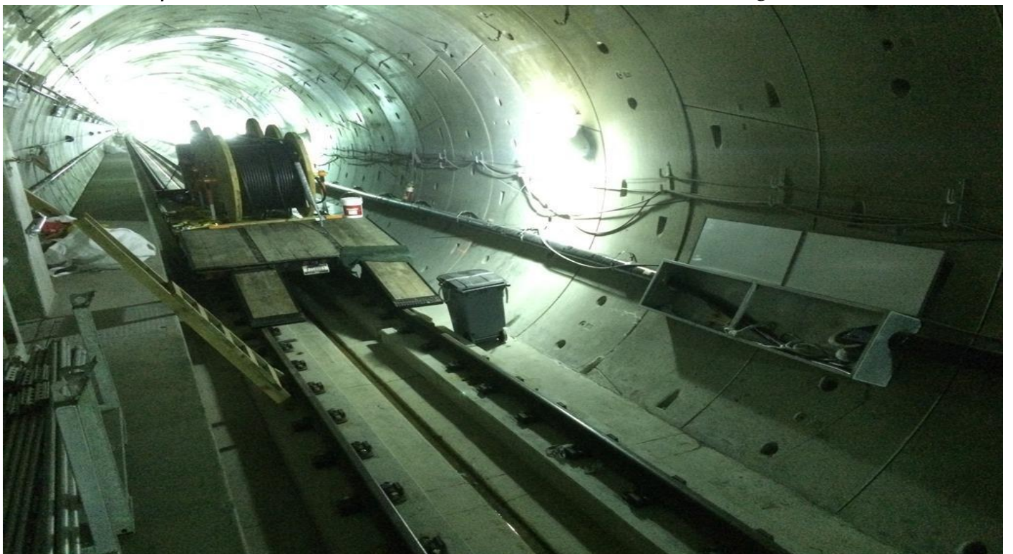
TUNNEL – Installation of electrical components at the SB tunnel between EXPO and MLK
