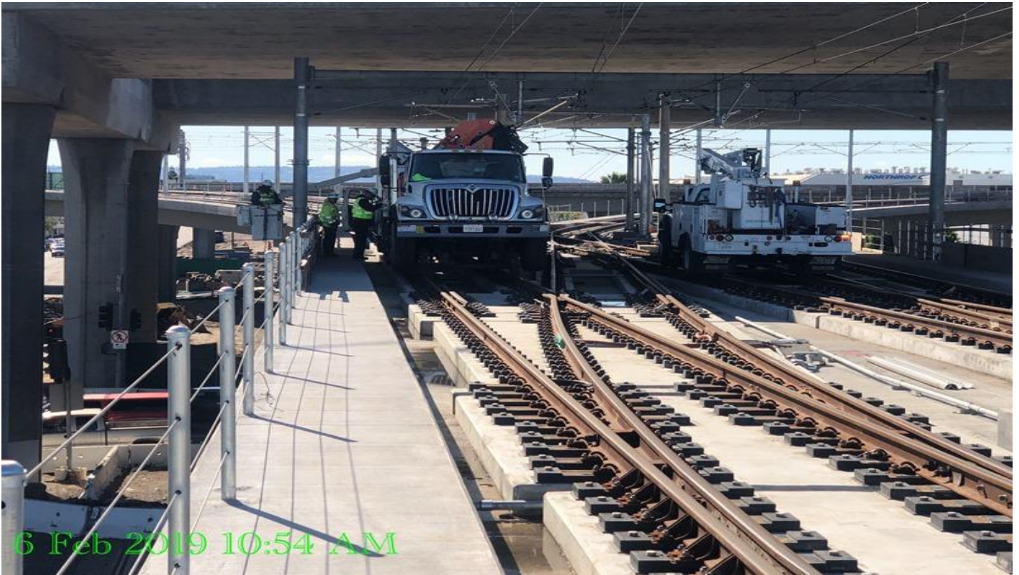
GREENLINE UNDERPASS - LKC lineman installation of EOS @ OCS Str. 1015E and 1015W at the Green Wye.
