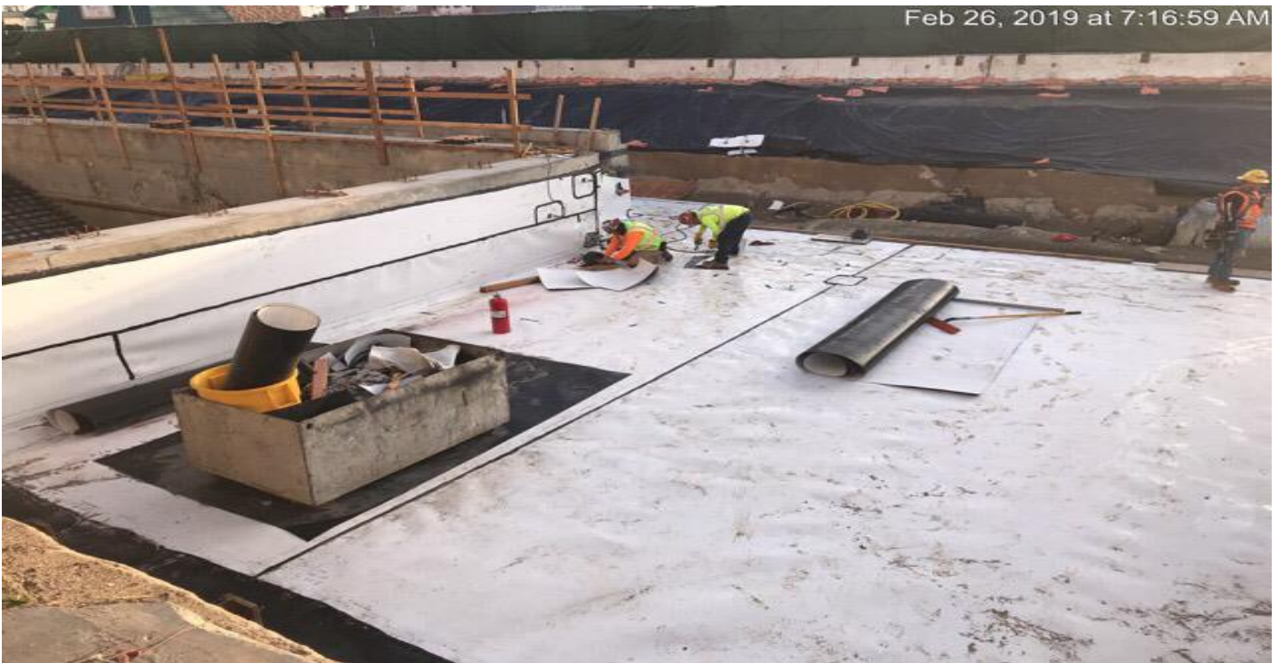
MARTIN LUTHER KING JR. STATION- Installation of waterproofing on the plaza roof.
