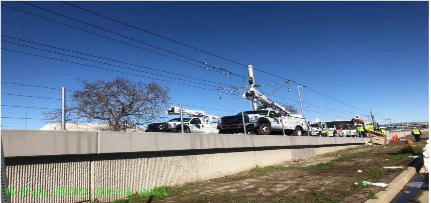
GREENLINE UNDERPASS- LKC lineman installation of EOS @ OCS Str. 1015E and 1015W. at the green wye.
