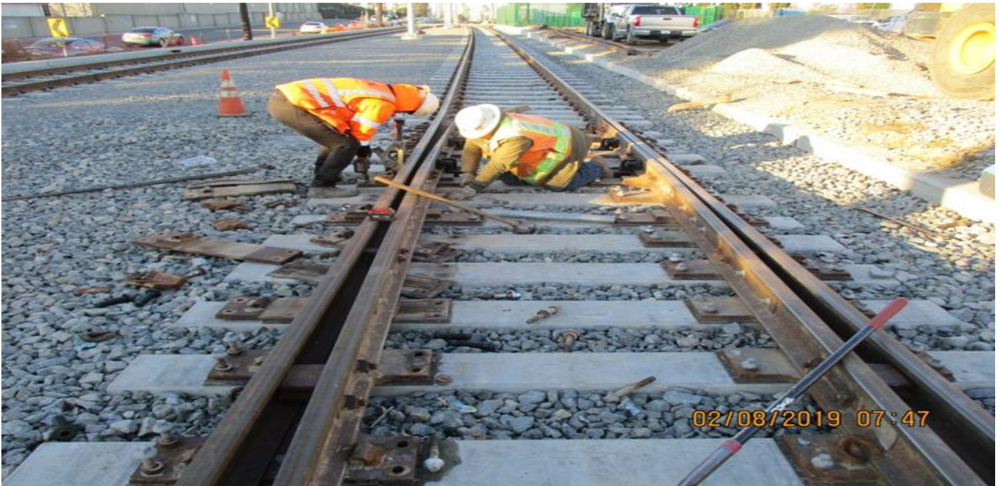
B1 GUIDEWAY - Replacing concrete tie inserts, patch concrete ties, and punch list at High st & West blvd.
