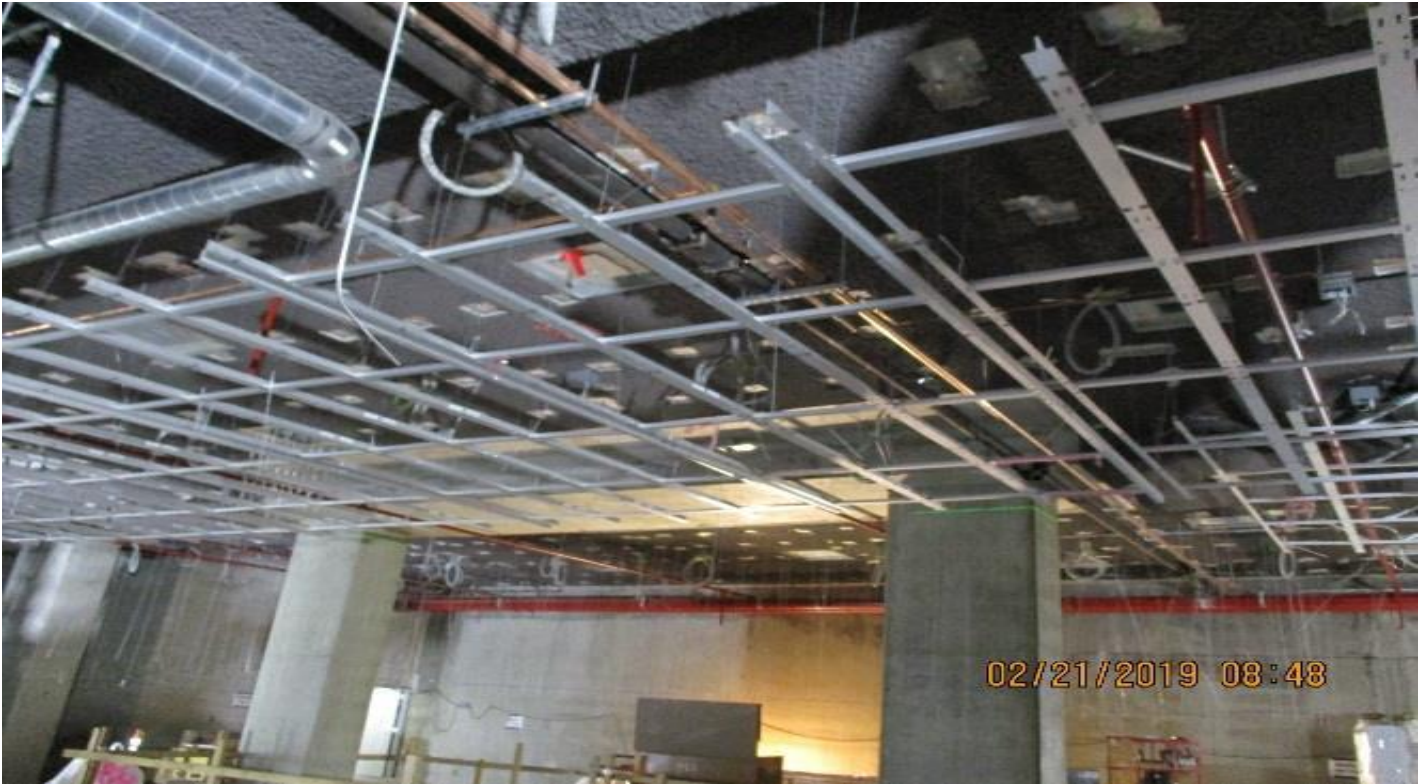
LEIMERT PARK STATION – Installation of metal ceiling at the Paid Area at the concourse.
