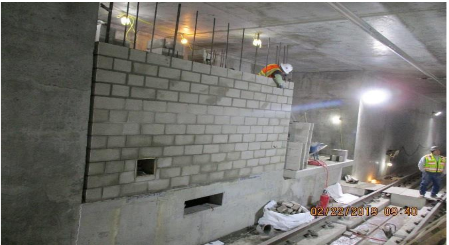
UG3- Installation of the CMU wall for the Radio room at the NB tunnel.
