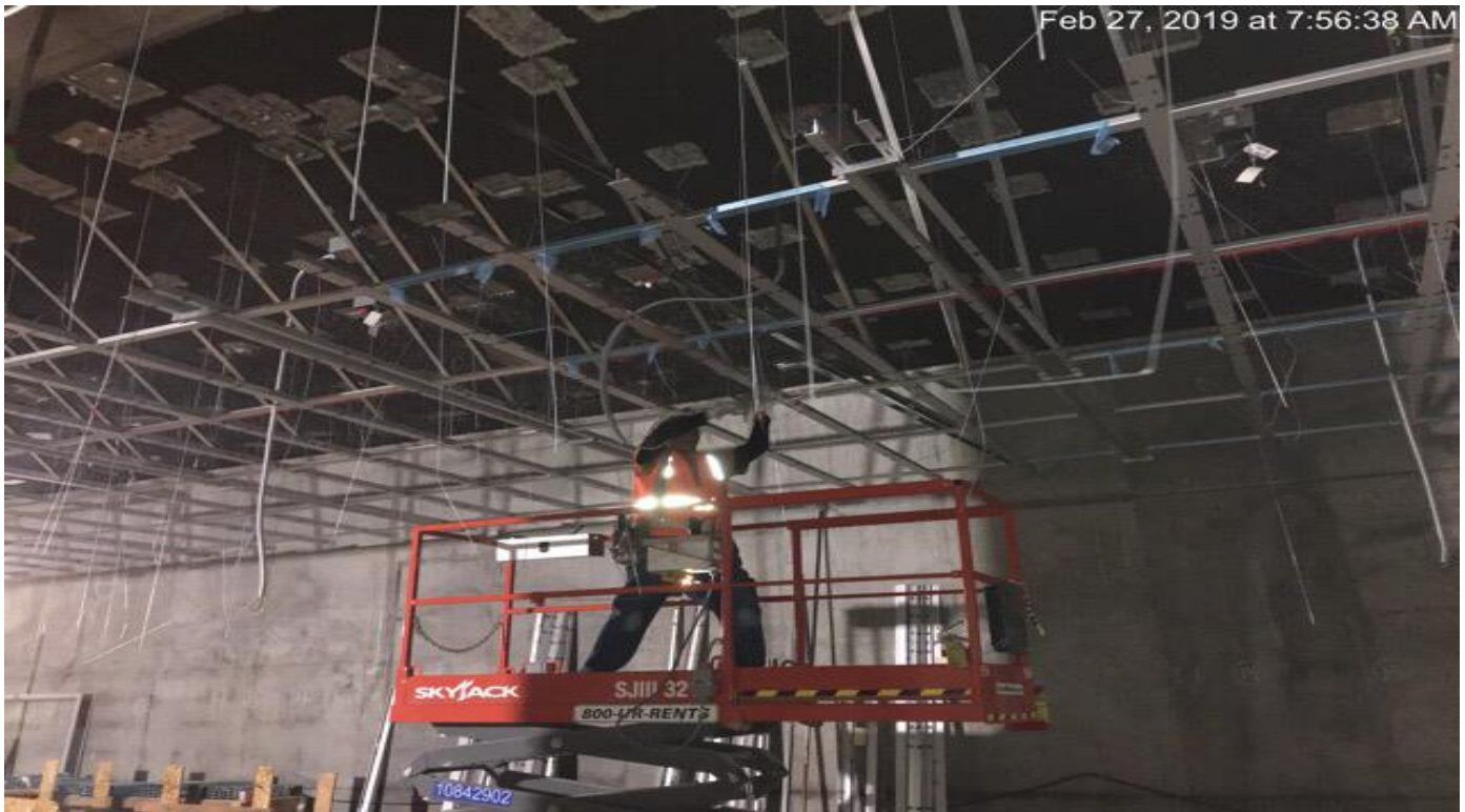
MARTIN LUTHER KING JR. STATION- Installation of the supports for the metal ceiling at the Paid Area at the concourse.
