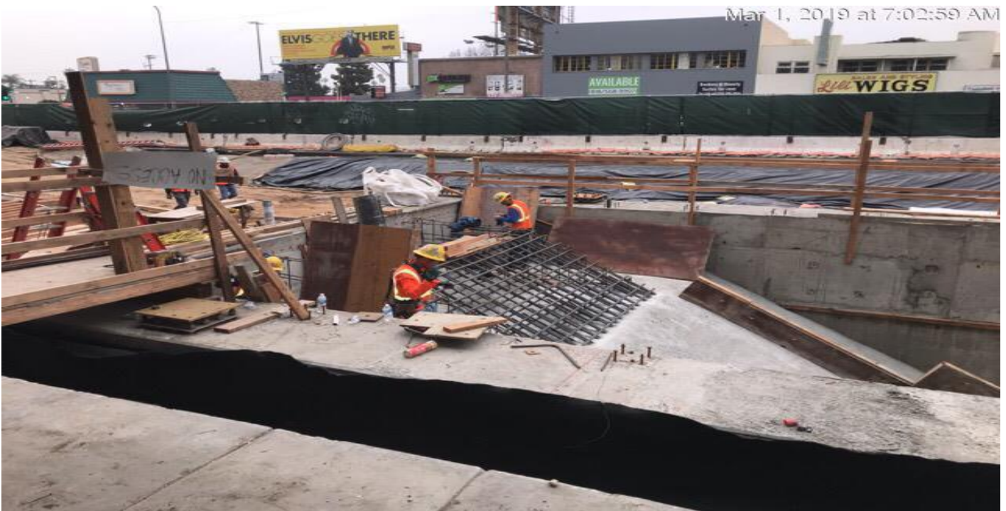
MARTIN LUTHER KING JR. STATION - Installation of staircase forms for plaza entrance.
