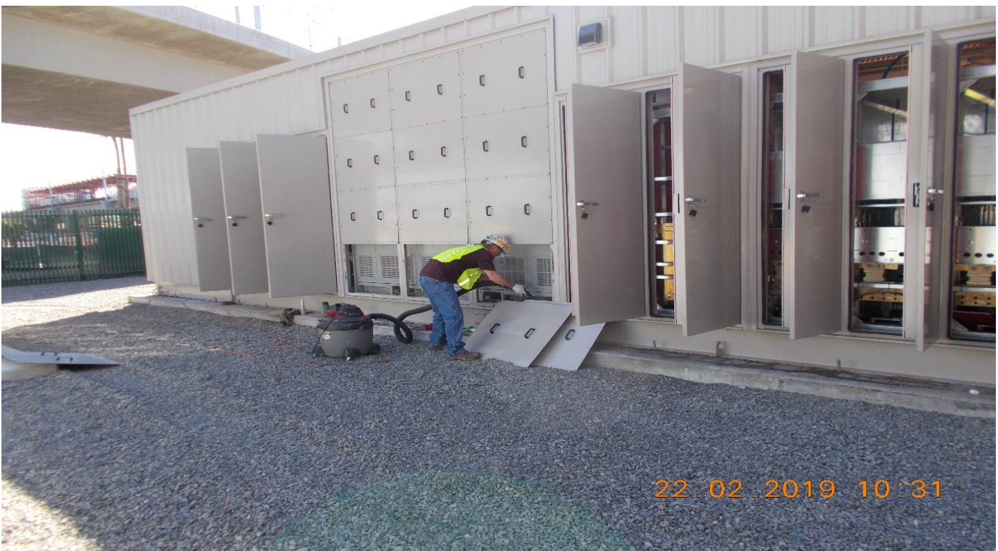
TPSS TPSS #1. NETE was re-doing the ground grid test without the TPSS enclosure grounds connected.
