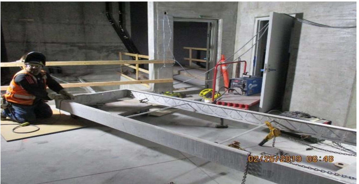
LEIMERT PARK STATION – Installation of equipment access hatch panels in the Emergency Ventilation Shaft/OTE Plenum South (C101).
