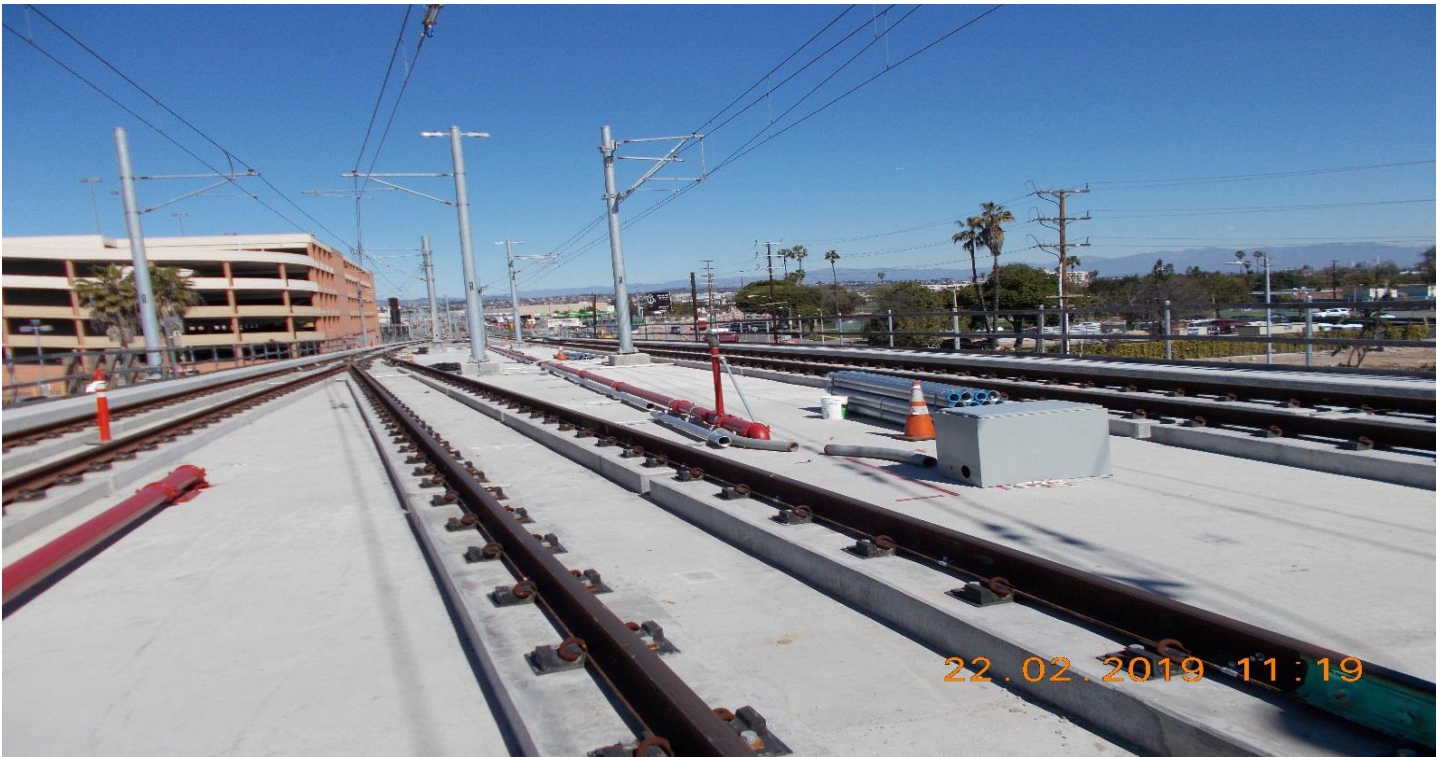
TPSS- TPSS #2. WSCC Electrical was working on Negative returns on the Guideway.
