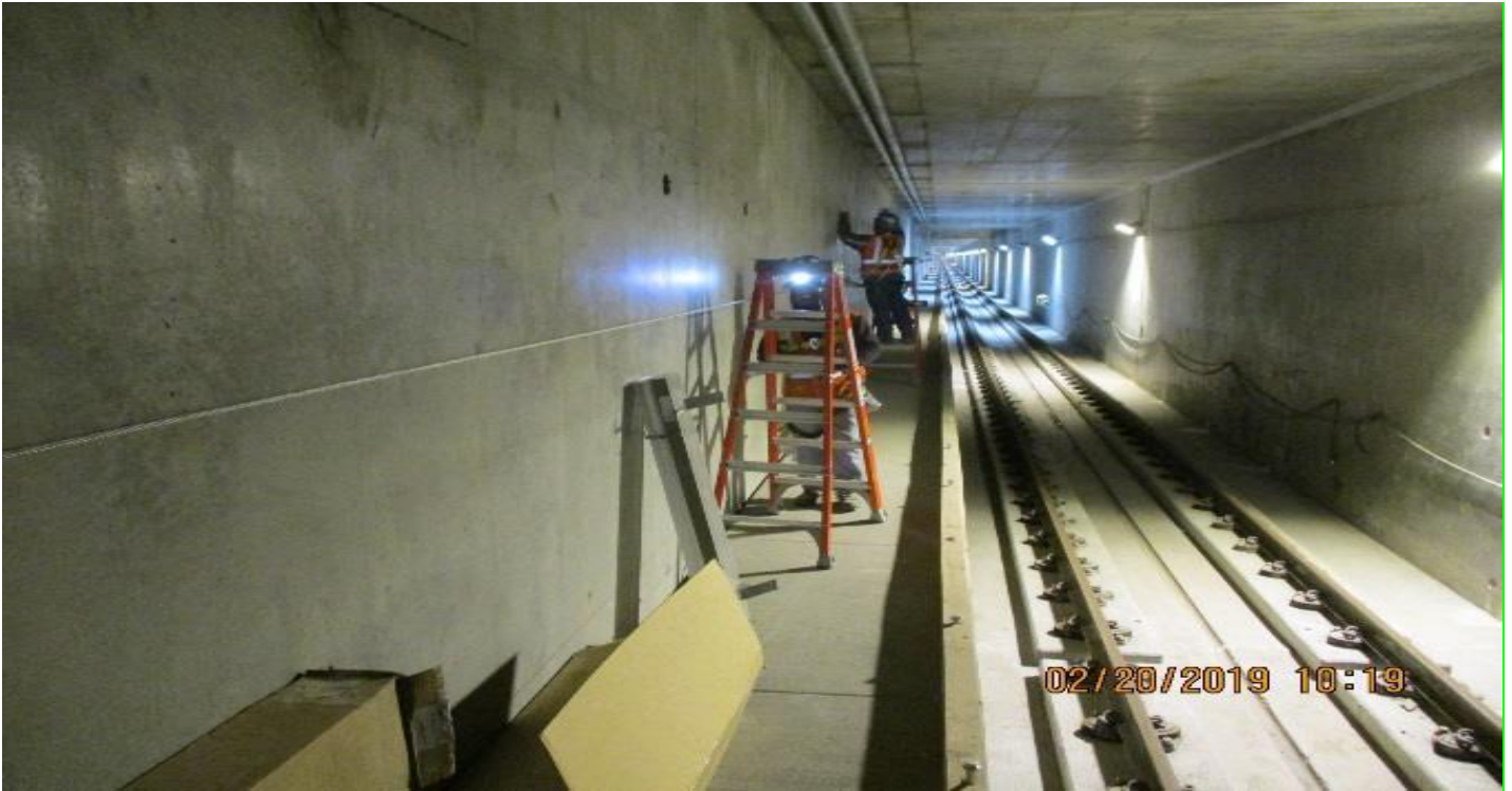
UG3- Installation of lighting fixtures and electrical components at the SB tunnel.
