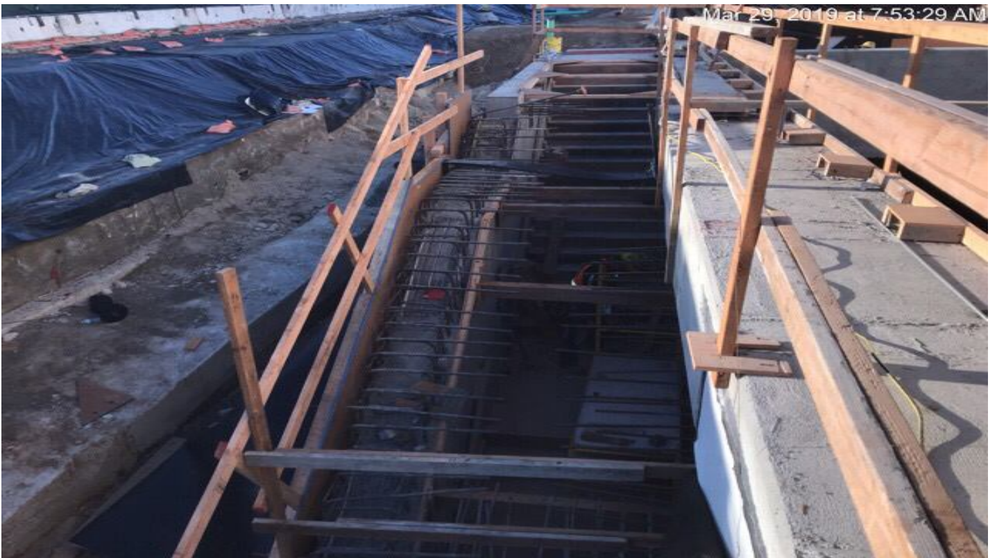
MARTIN LUTHER KING JR. STATION- Installation of falsework for Emergency Exit Stairs # 2 North.
