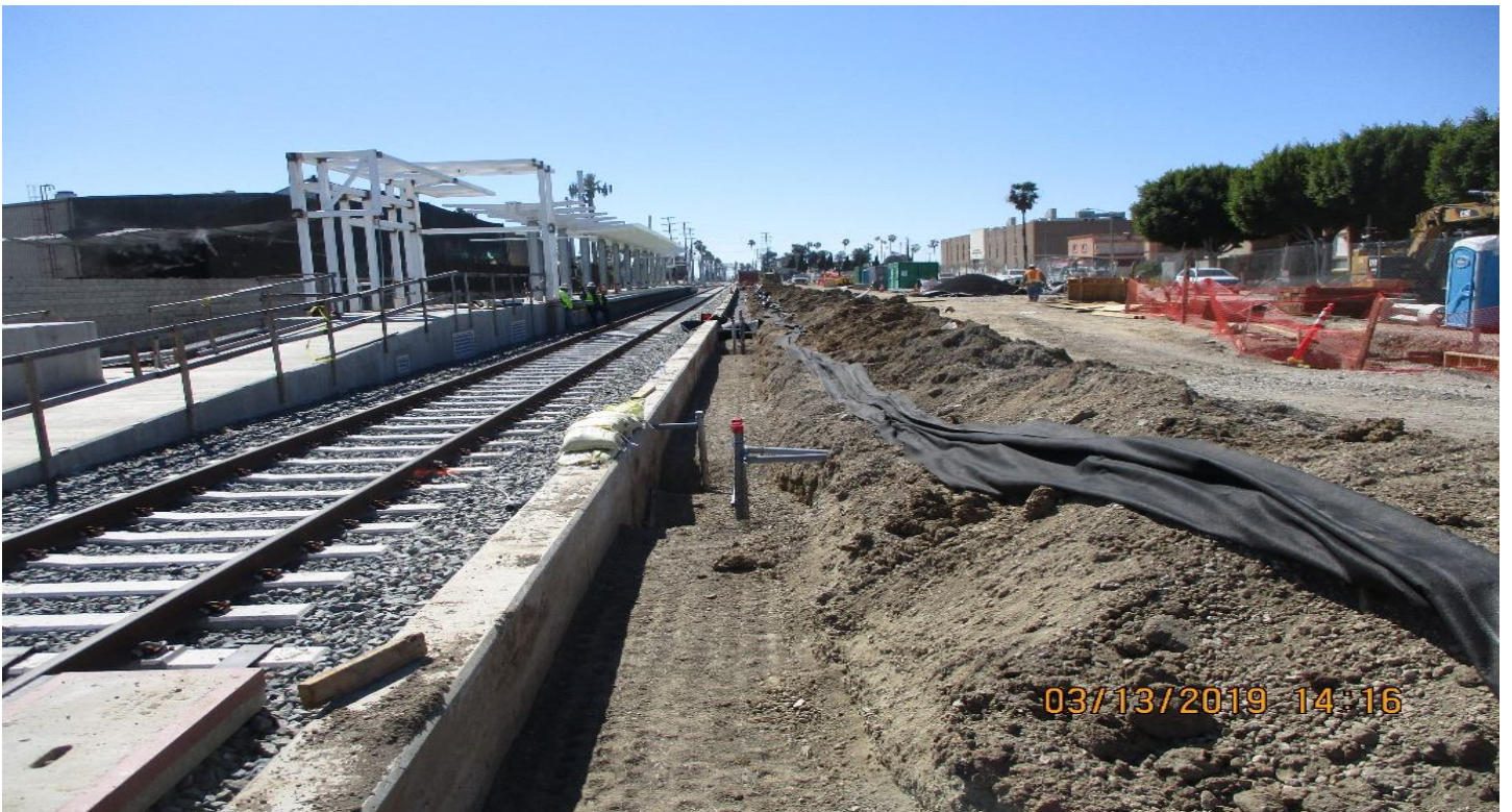
FAIRVIEW HEIGHTS STATION - Extending conduits on North Side of Southbound Ballast wall
