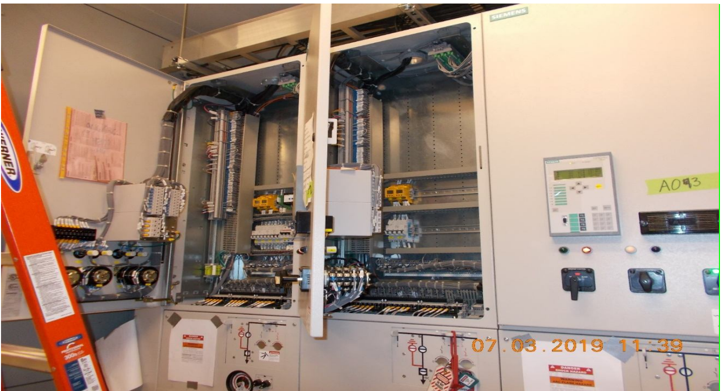
TPSS- AC switchgear upper cubicles.
