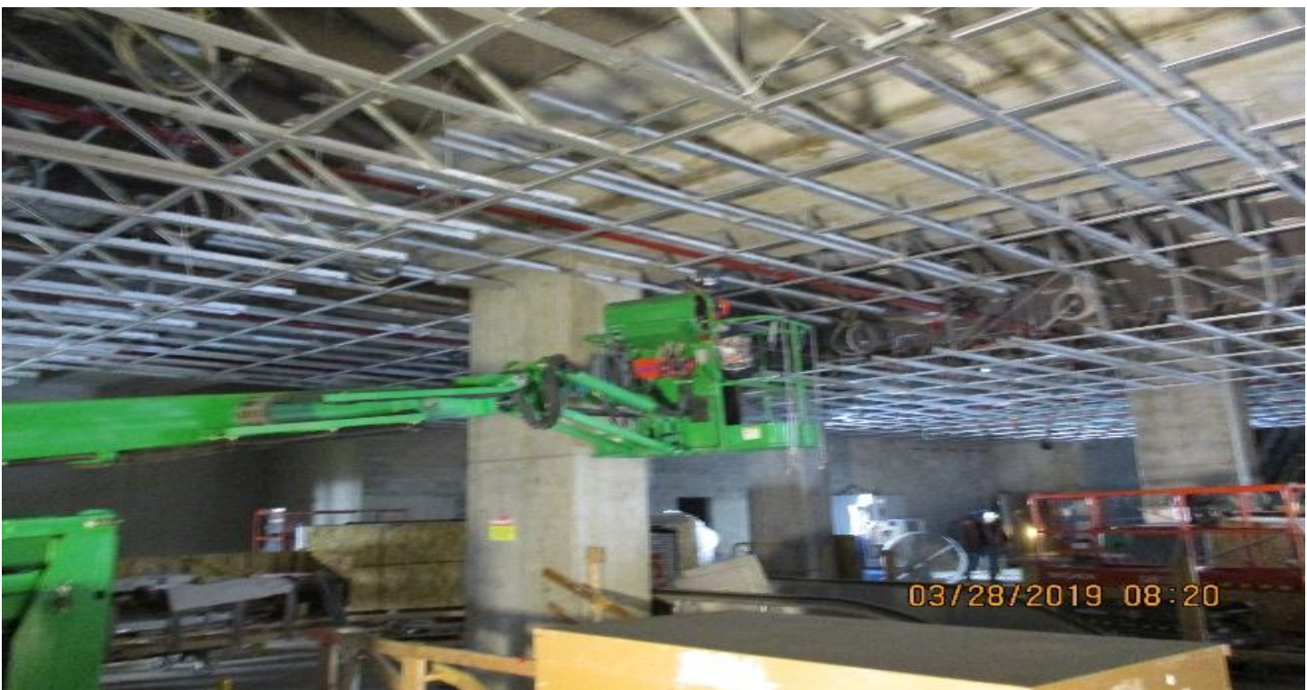
LEIMERT PARK STATION – Installation of the supports for the metal ceiling at the Concourse level.
