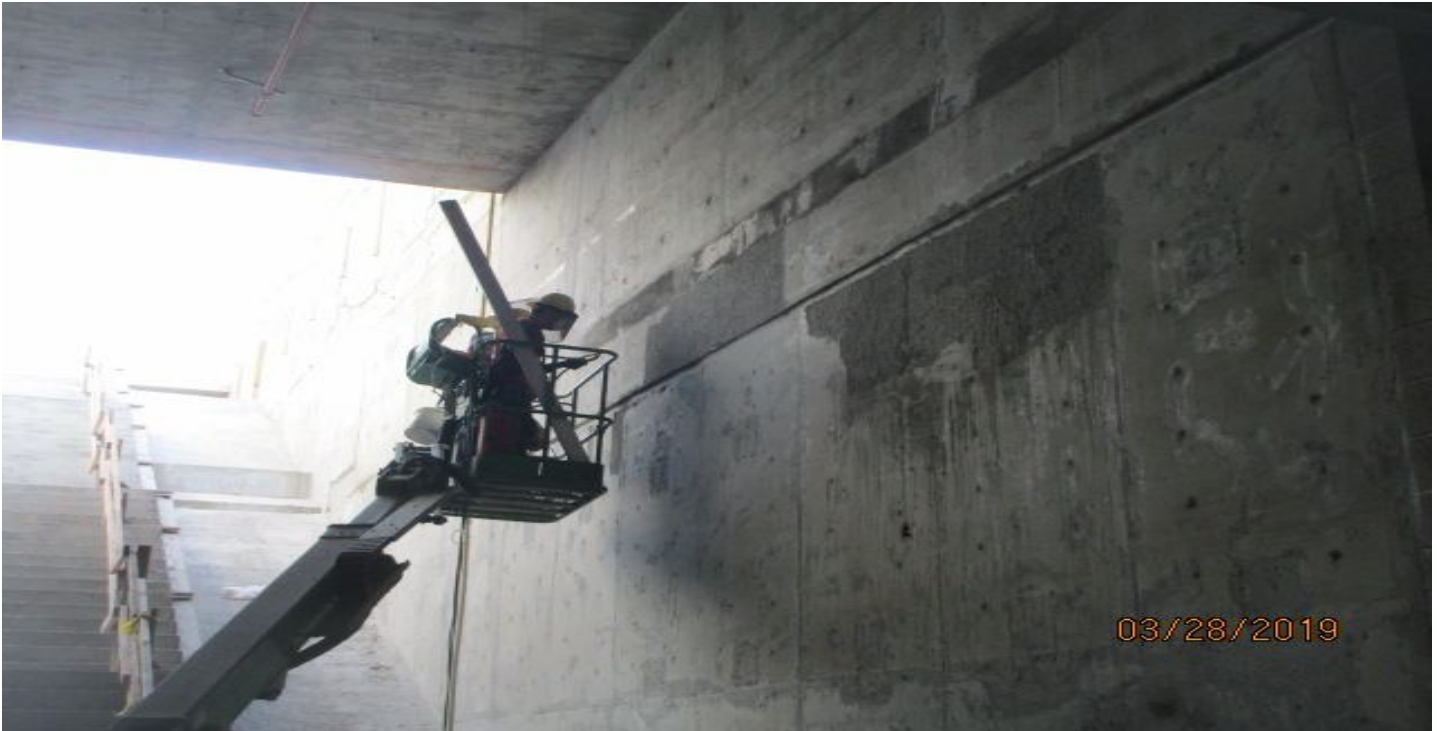
MARTIN LUTHER KING JR. STATION- Preparing wall joints at the concourse level.
