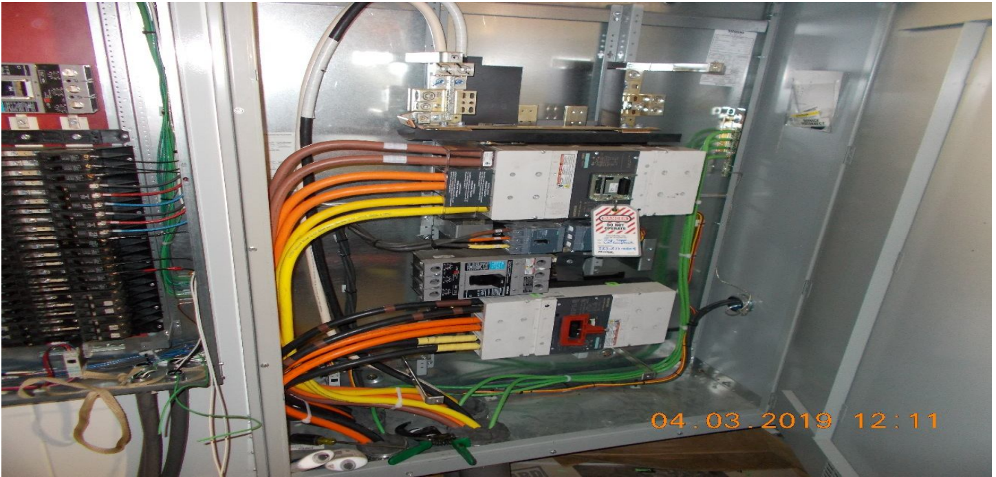
TPSS PP1 panel re-configured without generator feed.
