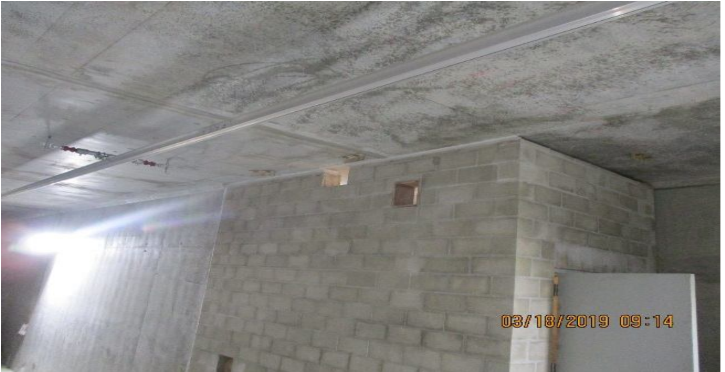
UG4 – Installation of fire caulk for the Radio room at the NB tunnel.
