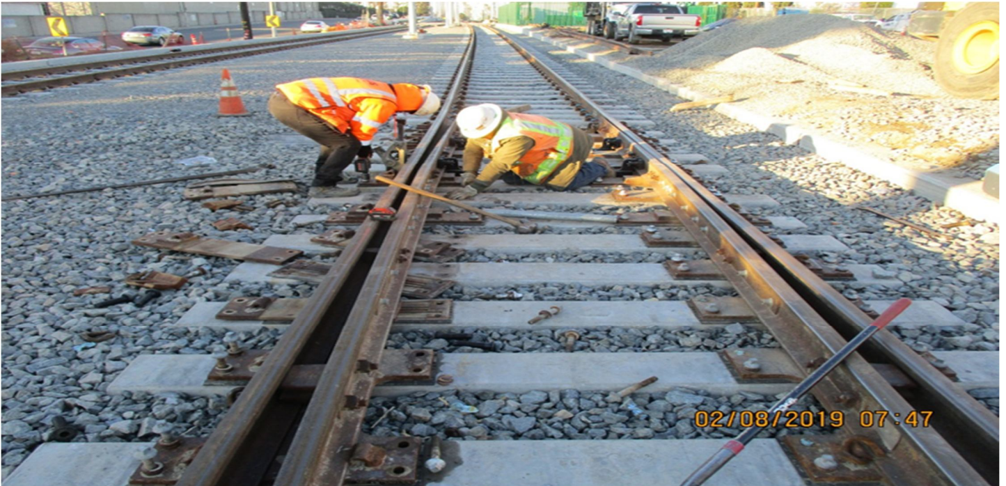
B1 GUIDEWAY - Replacing concrete tie inserts, patch concrete ties, and punch list at High st & West blvd.
