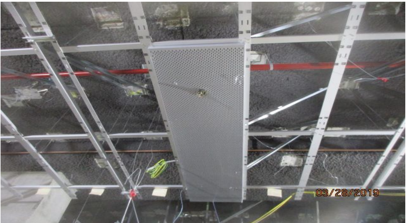
MARTIN LUTHER KING JR. STATION- Installation of the metal ceiling at the Concourse.
