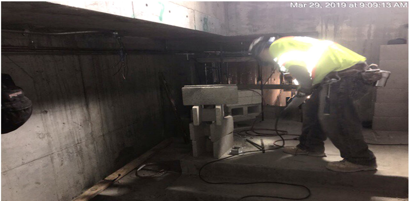
EXPOSITION/CRENSHAW STATION – Installed dowels for CMU wall M131 phase 2 at the Concourse level.
