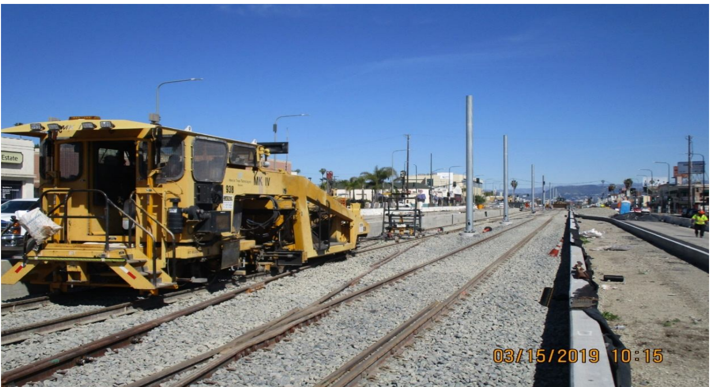
B2 GUIDEWAY 54 th to 57 th Streets – Rail surface, line, ballast tamping and dressing.
