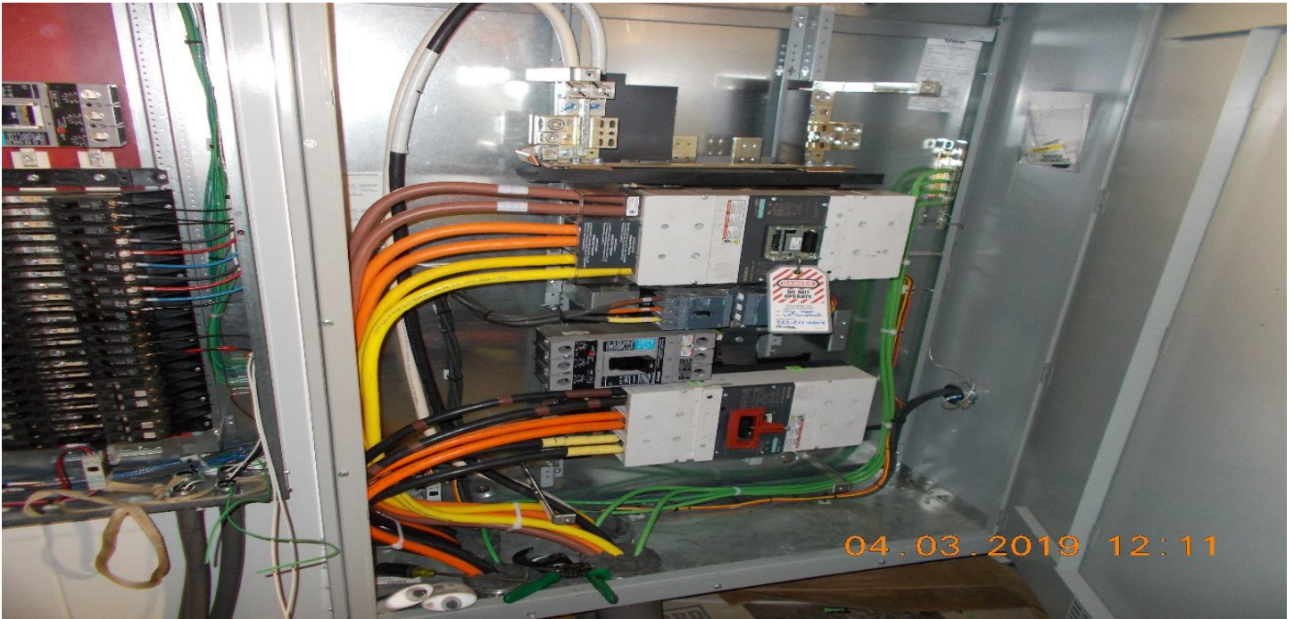
TPSS PP1 panel re-configured without generator feed.
