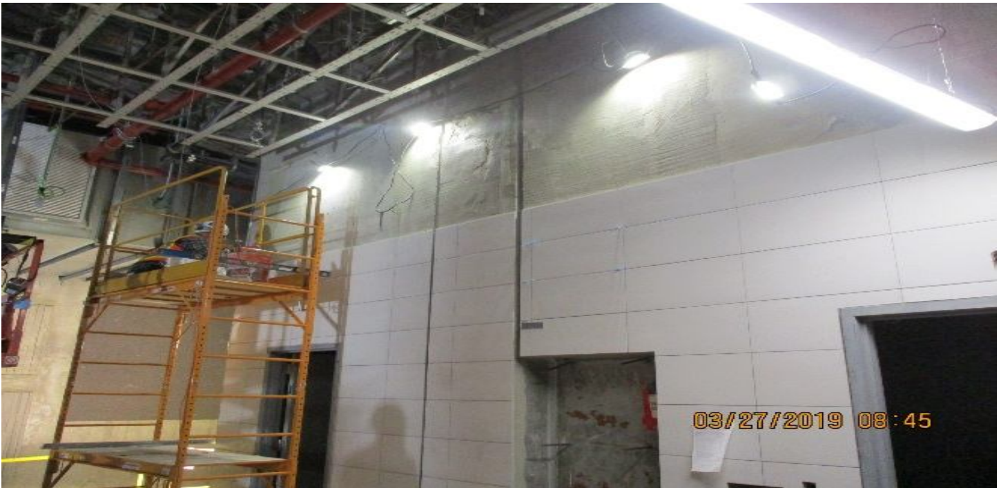
LEIMERT PARK STATION – Installation of ceramic tile at the Paid Area of the Concourse level.
