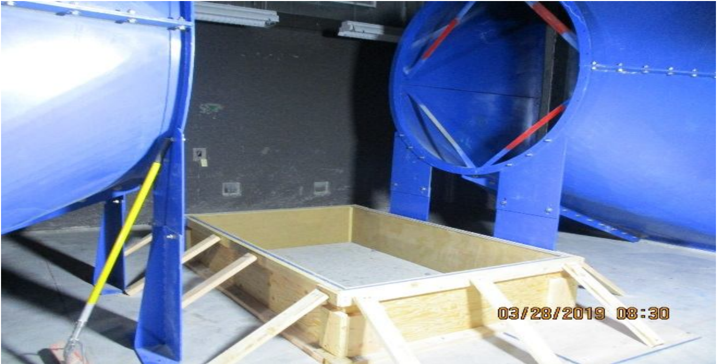
LEIMERT PARK STATION – Installation of formwork for the EVF equipment pad in the north and south Fan room.
