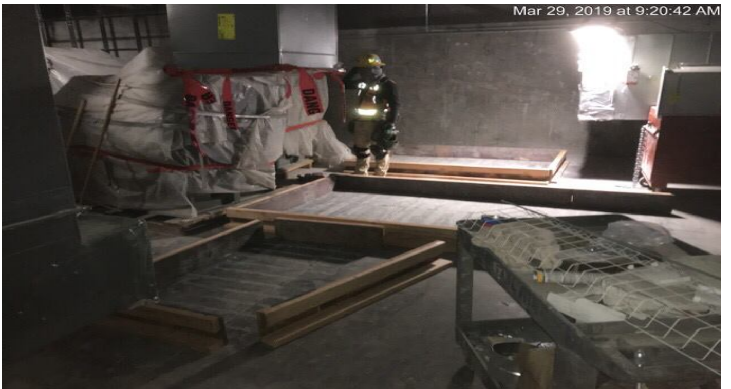
EXPOSITION/CRENSHAW STATION – Prepared formwork for equipment pads in Mechanical room North C146.
