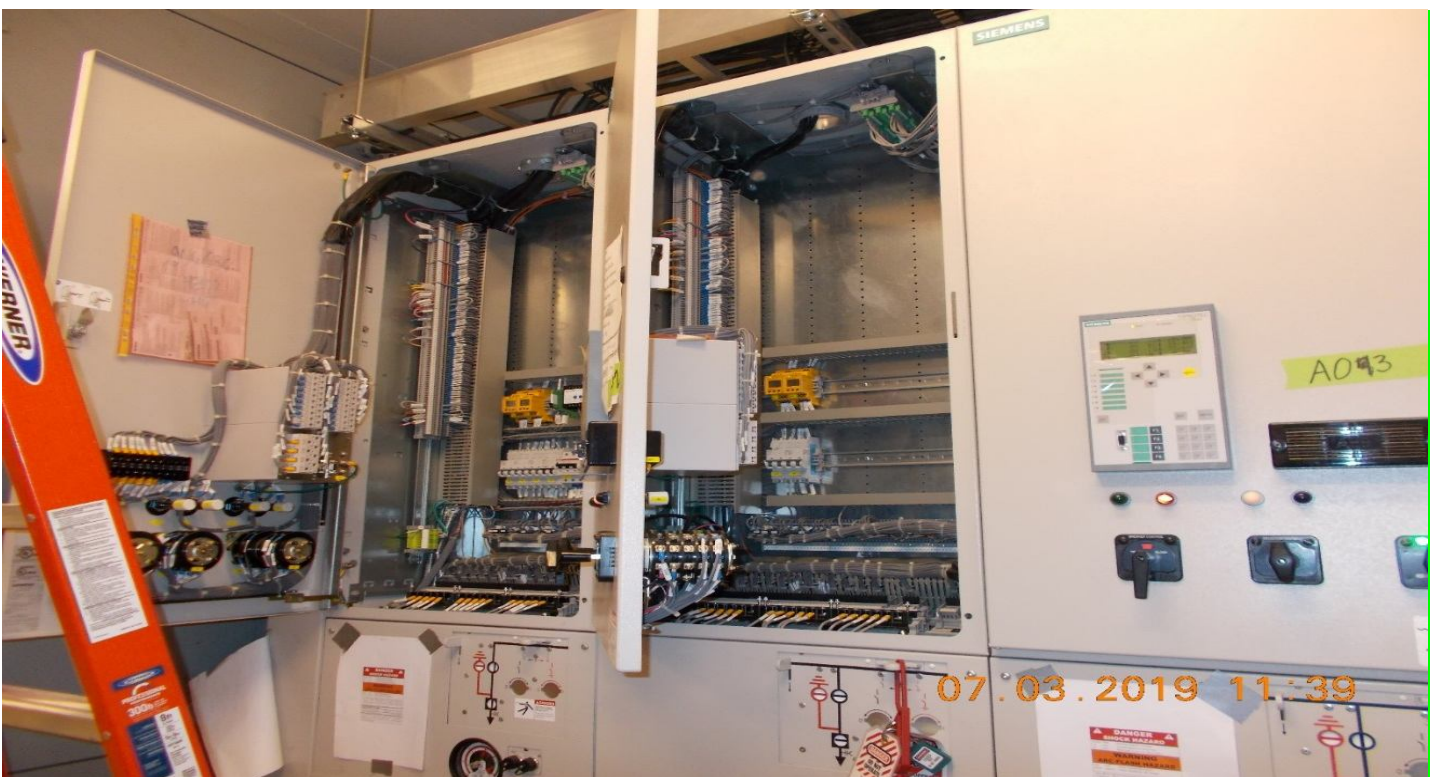
TPSS- AC switchgear upper cubicles.
