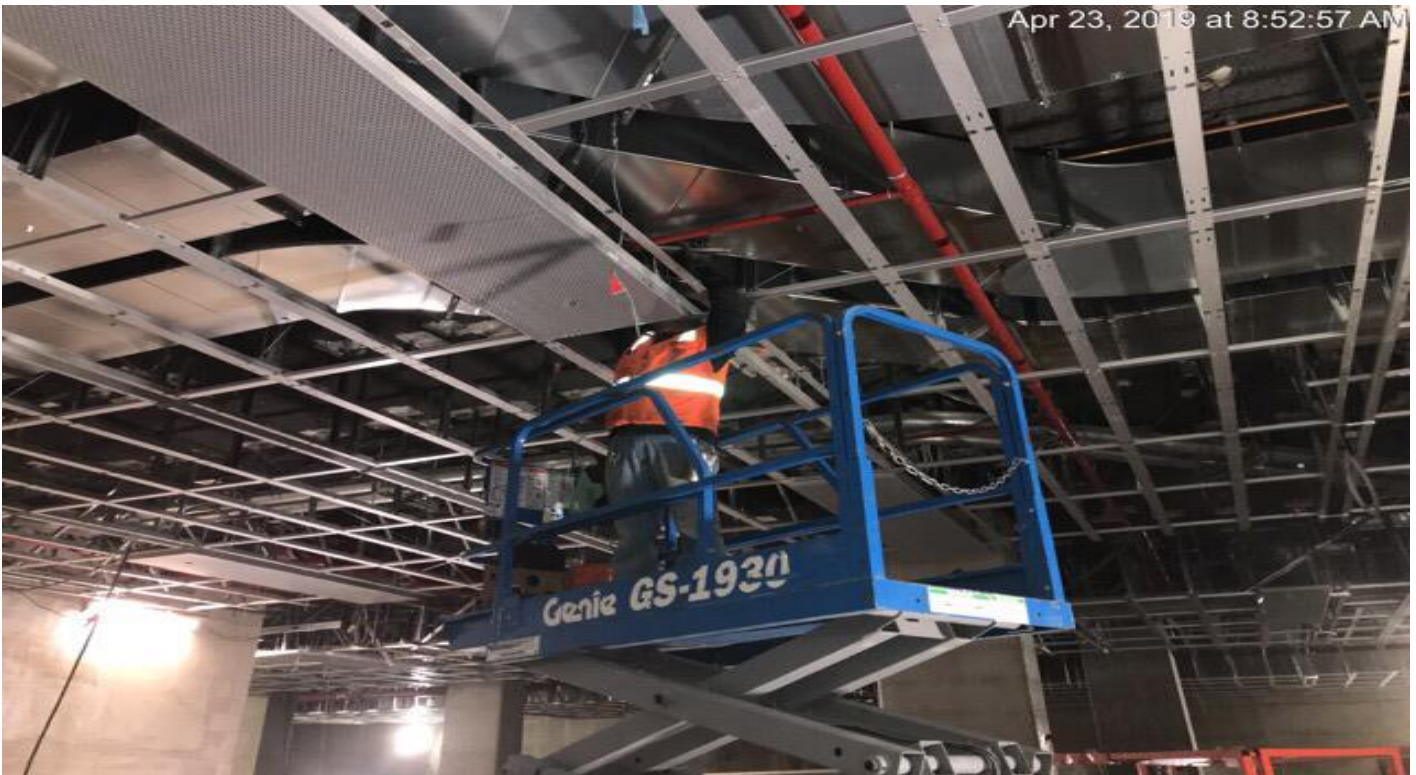
EXPOSITION/CRENSHAW STATION – Installation of the metal ceiling panel at the concourse public area.
