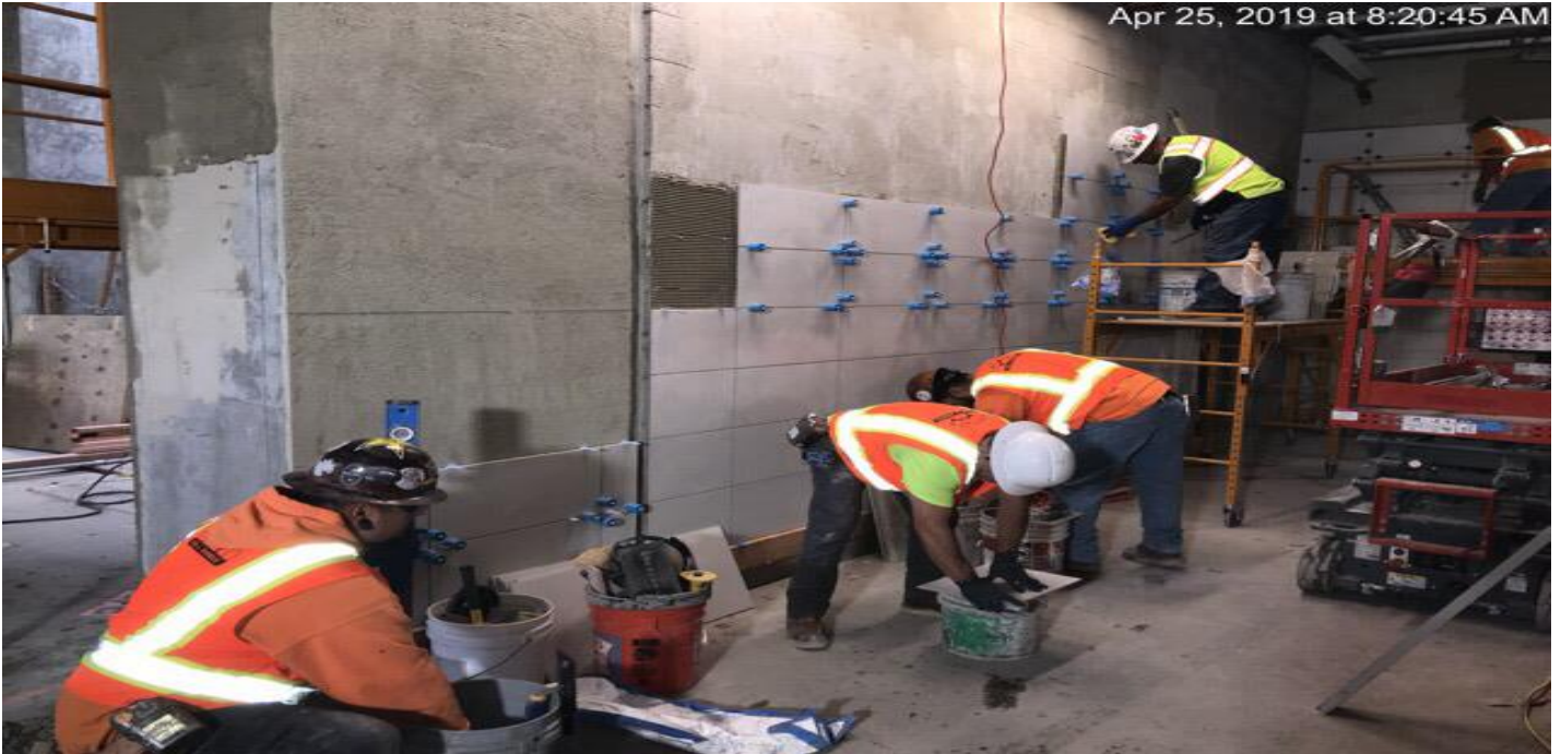
EXPOSITION/CRENSHAW STATION – Installation of ceramic tile at the concourse level public area.
