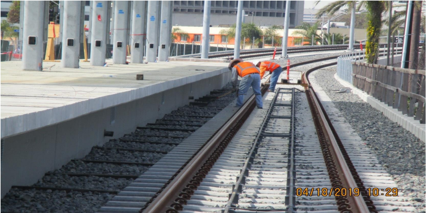
DOWNTOWN INGLEWOOD STATION- Guideway at La Brea Station install 6x6 treated lumber at conc ties.
