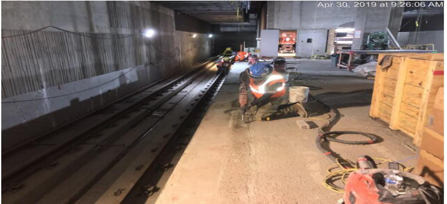
EXPOSITION/CRENSHAW STATION – Preparation of the platform edge for installation of the dielectric pad.
