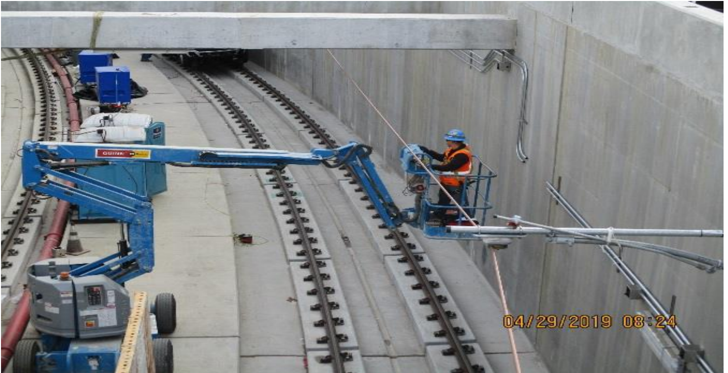
UG3- Installation of conduit for walkway lighting along the wall at the south portal.
