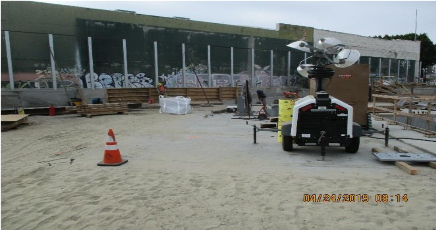
LEIMERT PARK STATION – Removal of formwork from the green screen wall at the southeastern end of the station yard.
