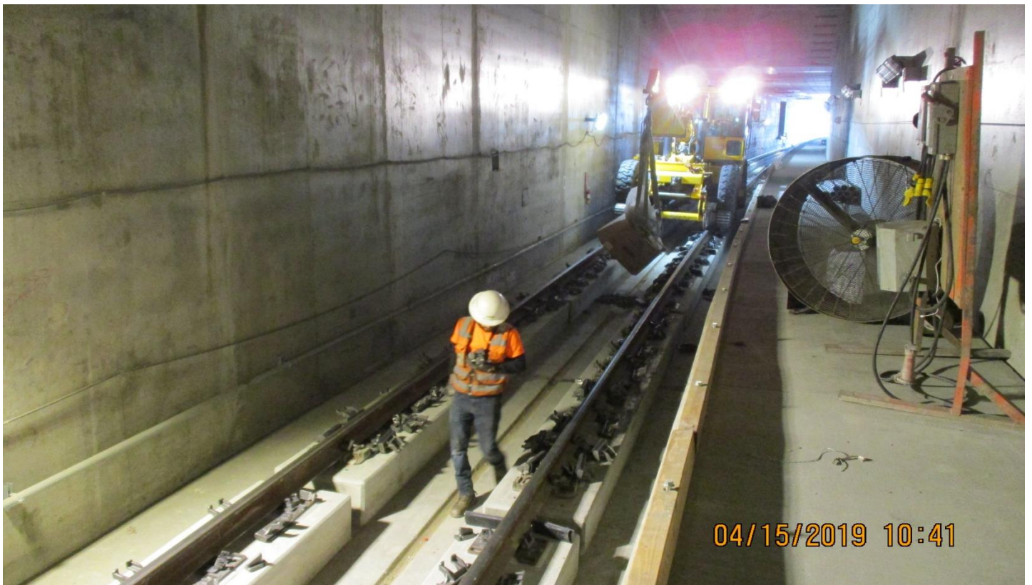
TUNNEL – STA 372+71 to 377+40 layout of very high resilient direct fixation rail fasteners.
