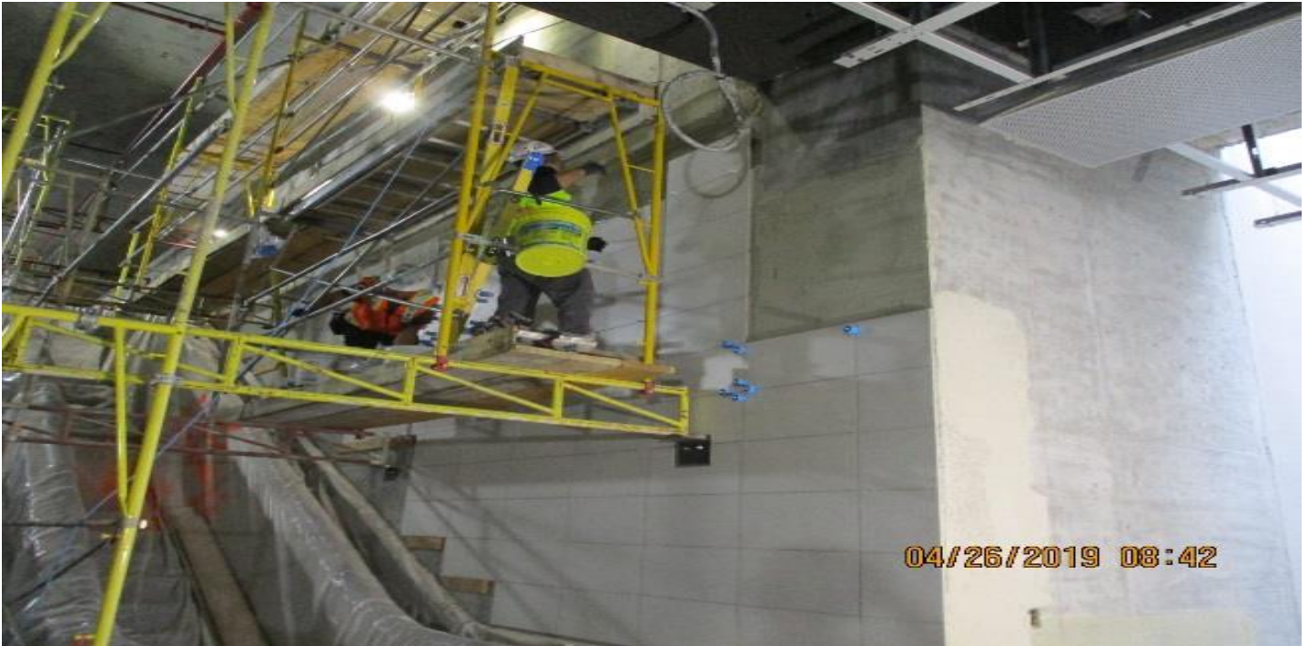
LEIMERT PARK STATION – Installation of ceramic tile at the entrance stairway walls.
