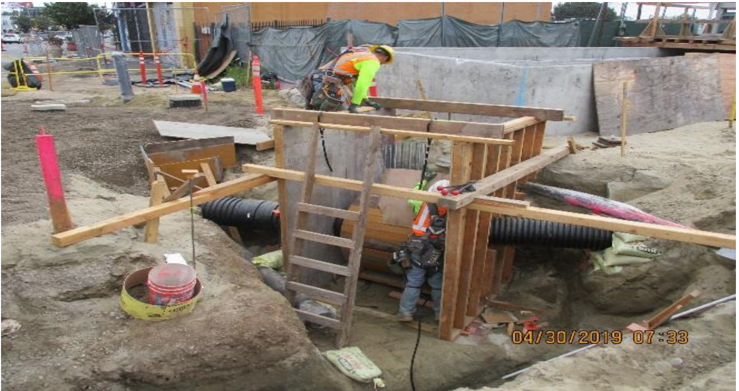
LEIMERT PARK STATION – Pipe relocation for the oil water separator at the station yard.
