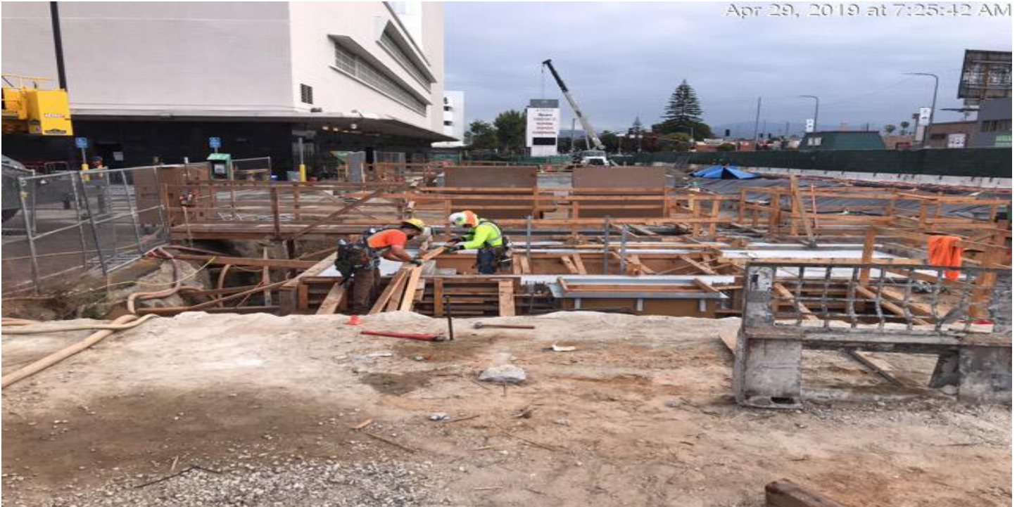
MARTIN LUTHER KING JR. STATION- Construction of the ramp and the entrance to Emergency Exit 2 South.
