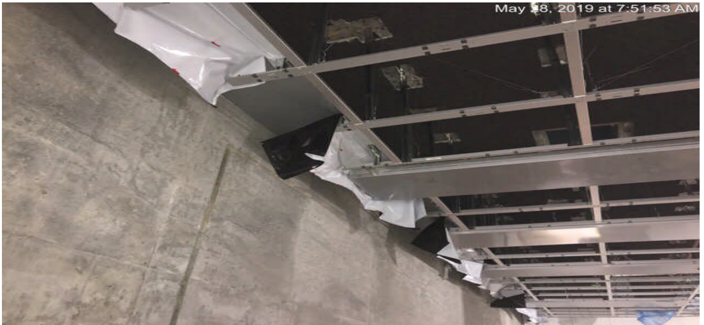
MARTIN LUTHER KING JR. STATION- Installation of top reflector plates at the concourse level.
