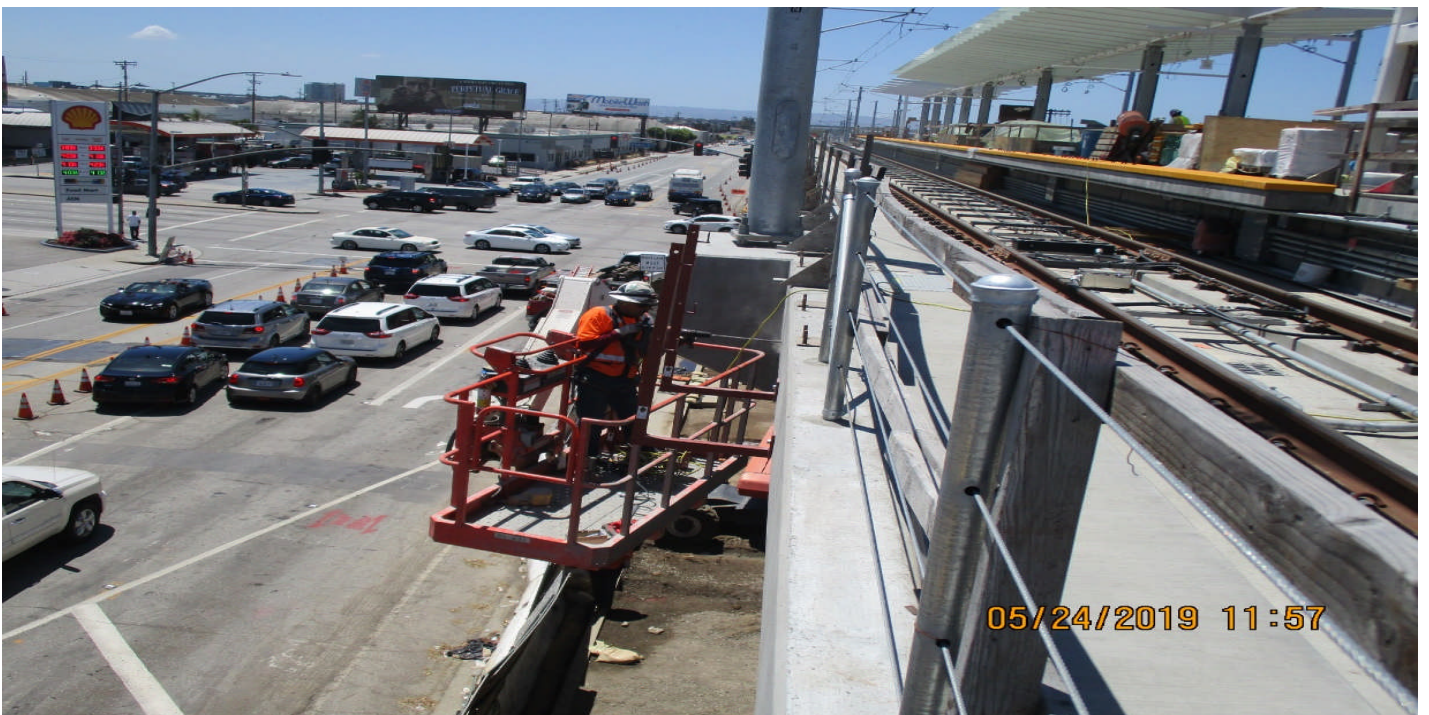
AVIATION/CENTURY- A Guideway at Aviation-Century UP NB coping slab overhang bracket install.
