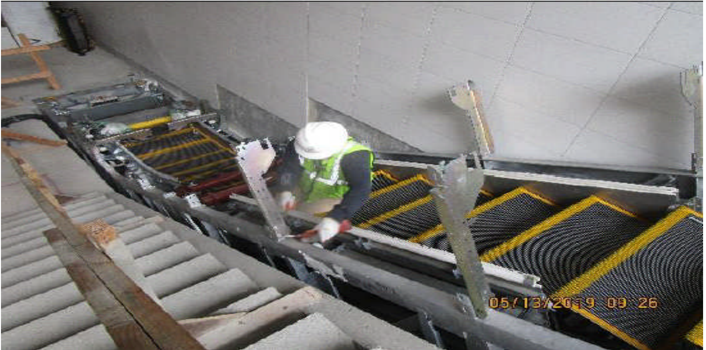
MARTIN LUTHER KING JR. STATION- Installation of Escalator 1 & 2 at plaza to concourse level.
