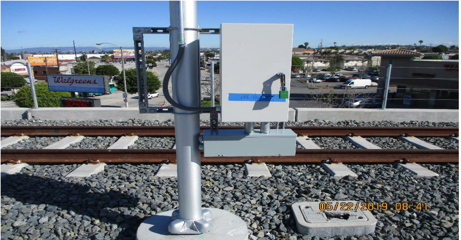
DOWNTOWN INGLEWOOD STATION- Camera Pole and CIC on East approach to the La Brea Bridge.
