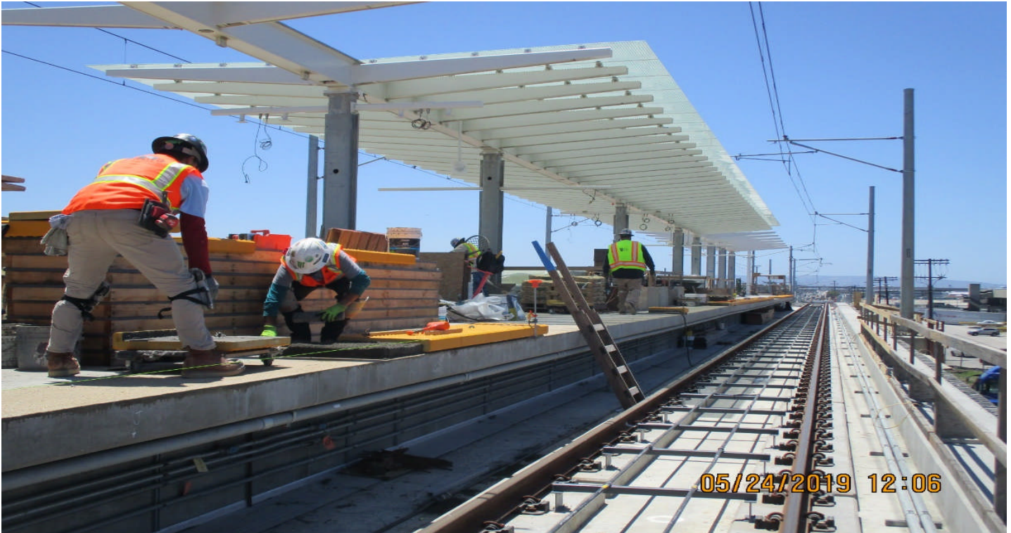
AVIATION/CENTURY- A Guideway at Aviation-Century UP NB coping slab overhang bracket install.
