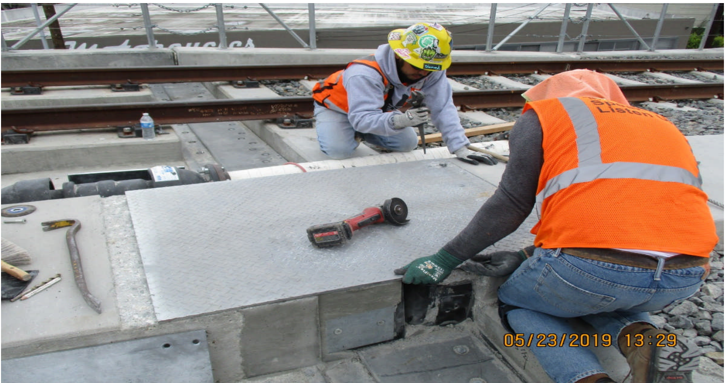
405 BRIDGE - A Guideway at 405 UP About 5 stripping of electrical duct bank and complete repair at JSA.
