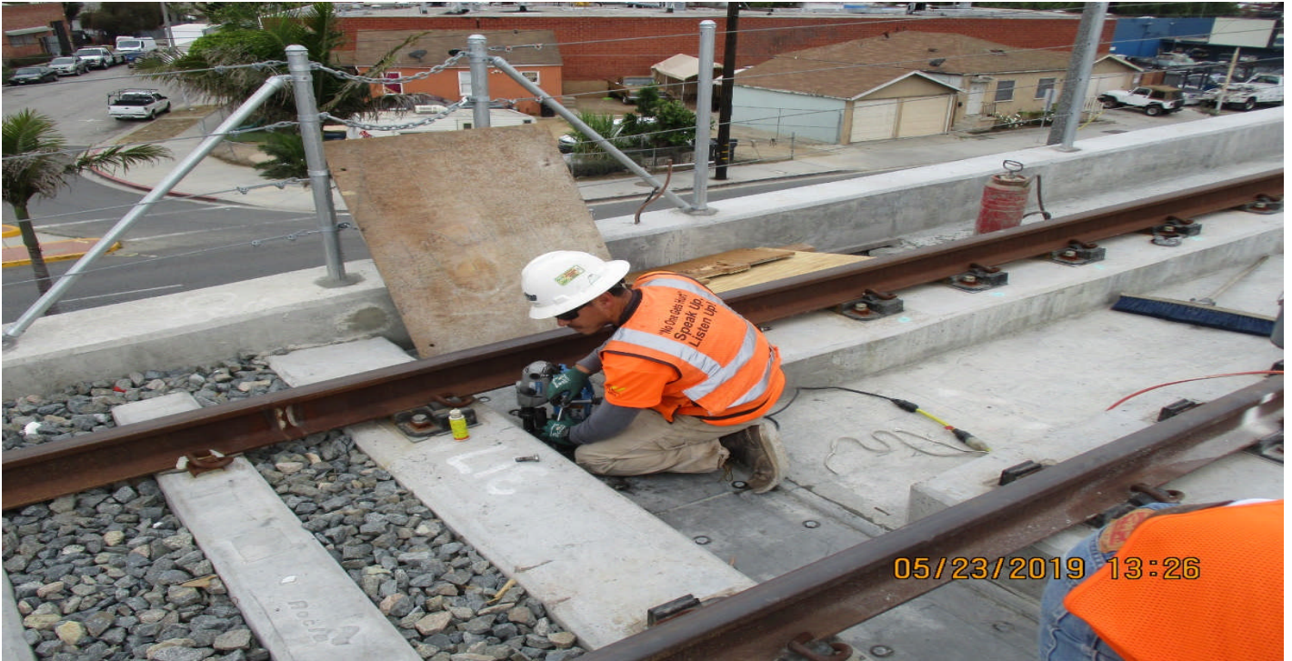
405 BRIDGE - A Guideway at 405 UP About 5 stripping of electrical duct bank and complete repair at JSA.
