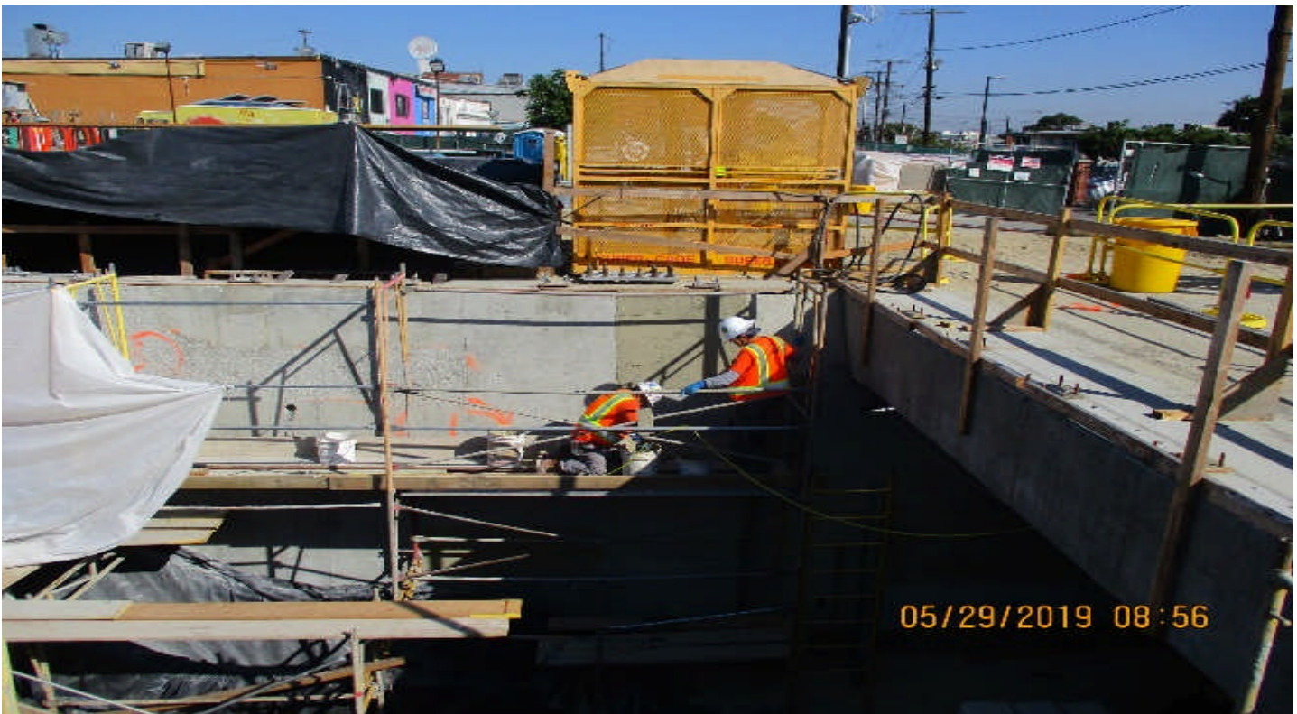
LEIMERT PARK STATION – Tile installation from mid landing to plaza at entrance stairs #1.
