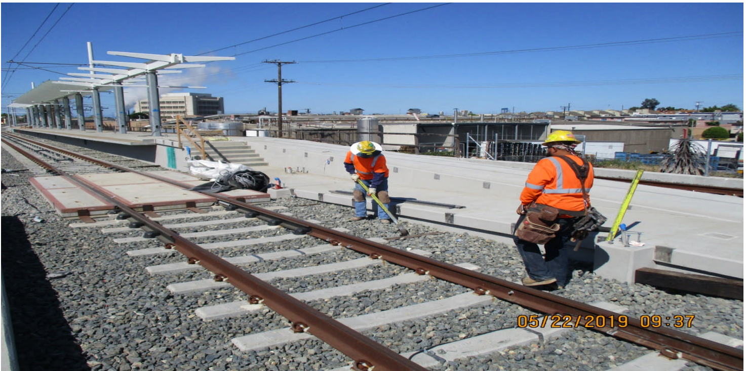
DOWNTOWN INGLEWOOD STATION- A Guideway at La Brea Station removal of 6x6 treated lumber.
