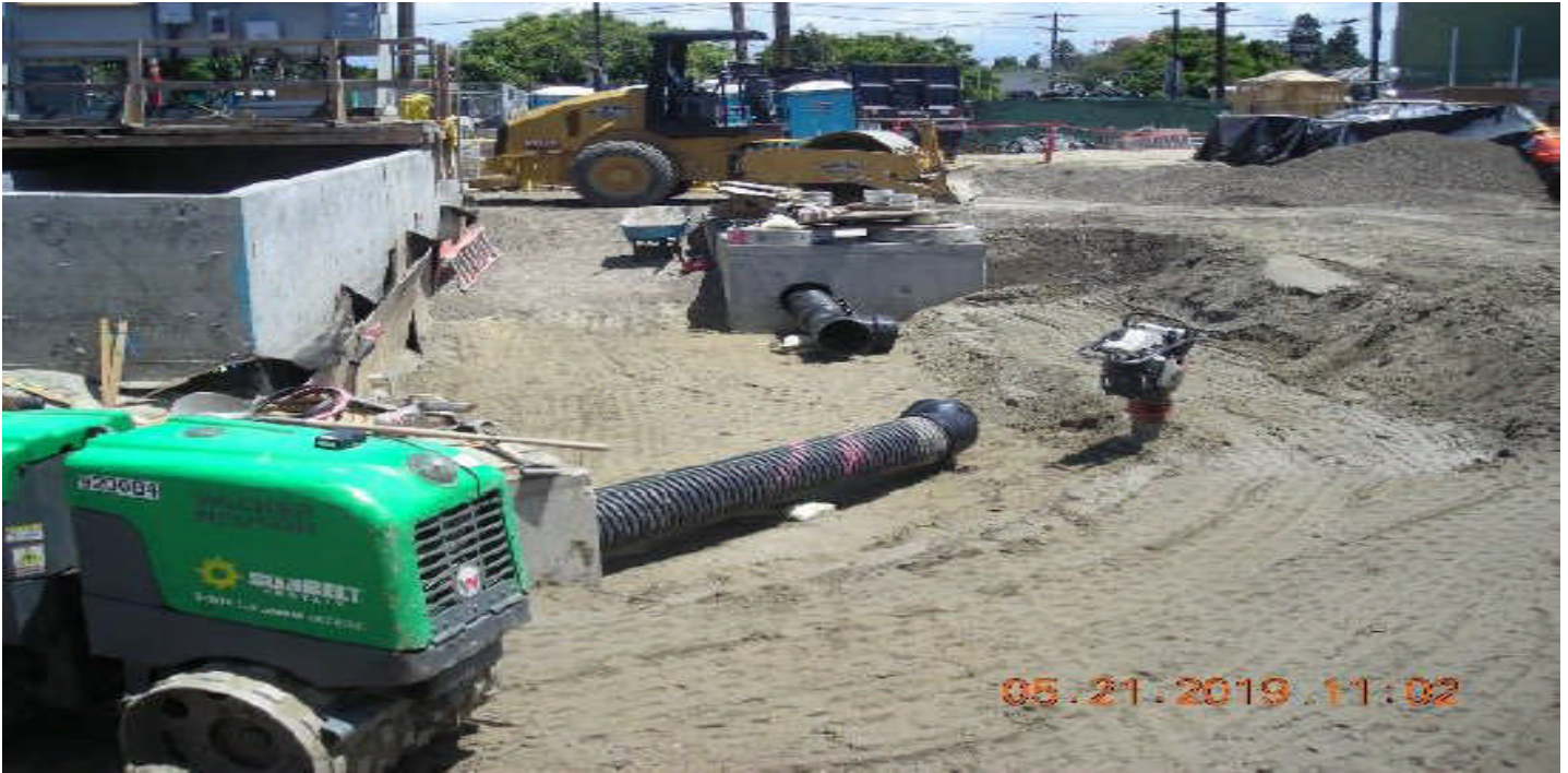
LEIMERT PARK STATION – Backfill w/ storm drain for oil/water separator at station yard.
