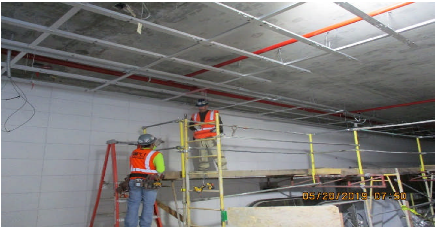
LEIMERT PARK STATION – Installation of metal ceiling grid at the concourse level.
