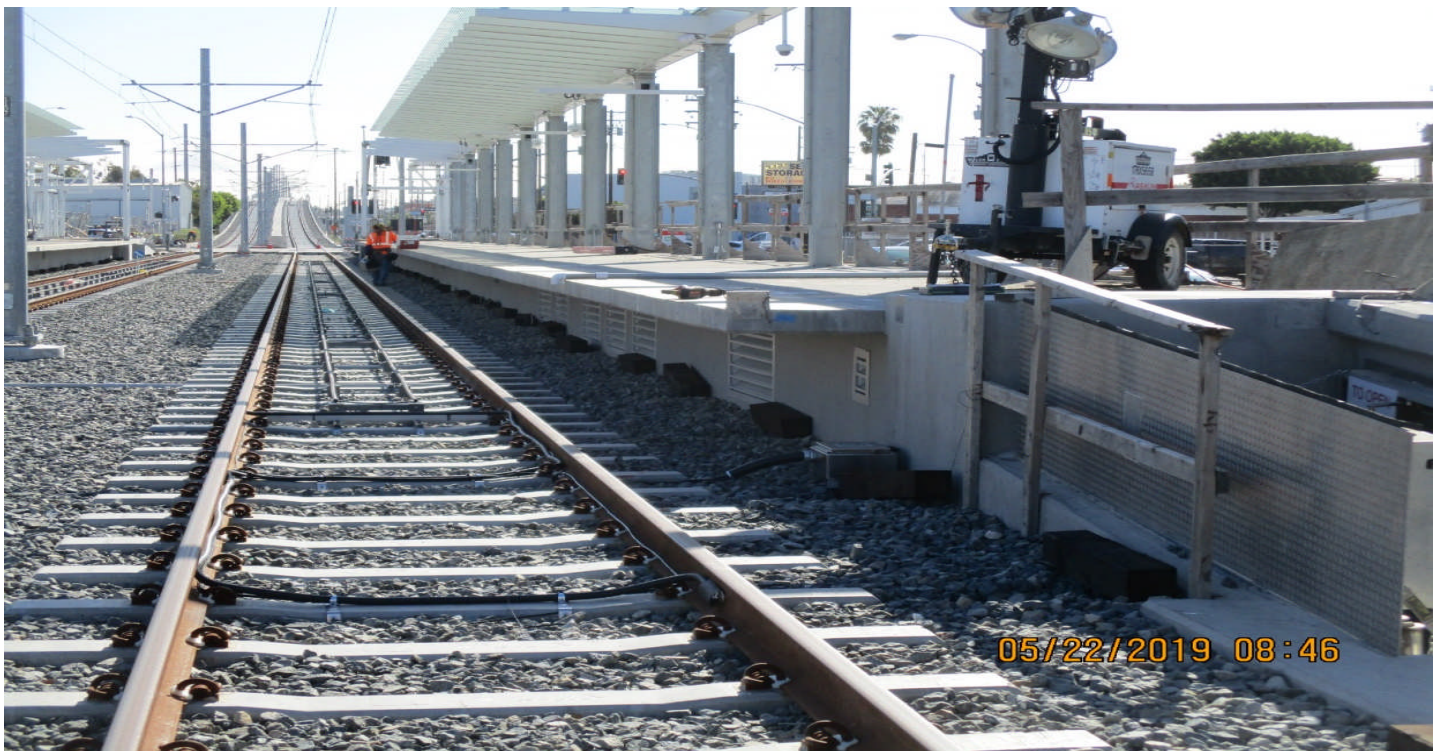
FLORENCE/HINDRY - A Guideway at Hindry Station removal of 6x6 treated lumber along both tracks.
