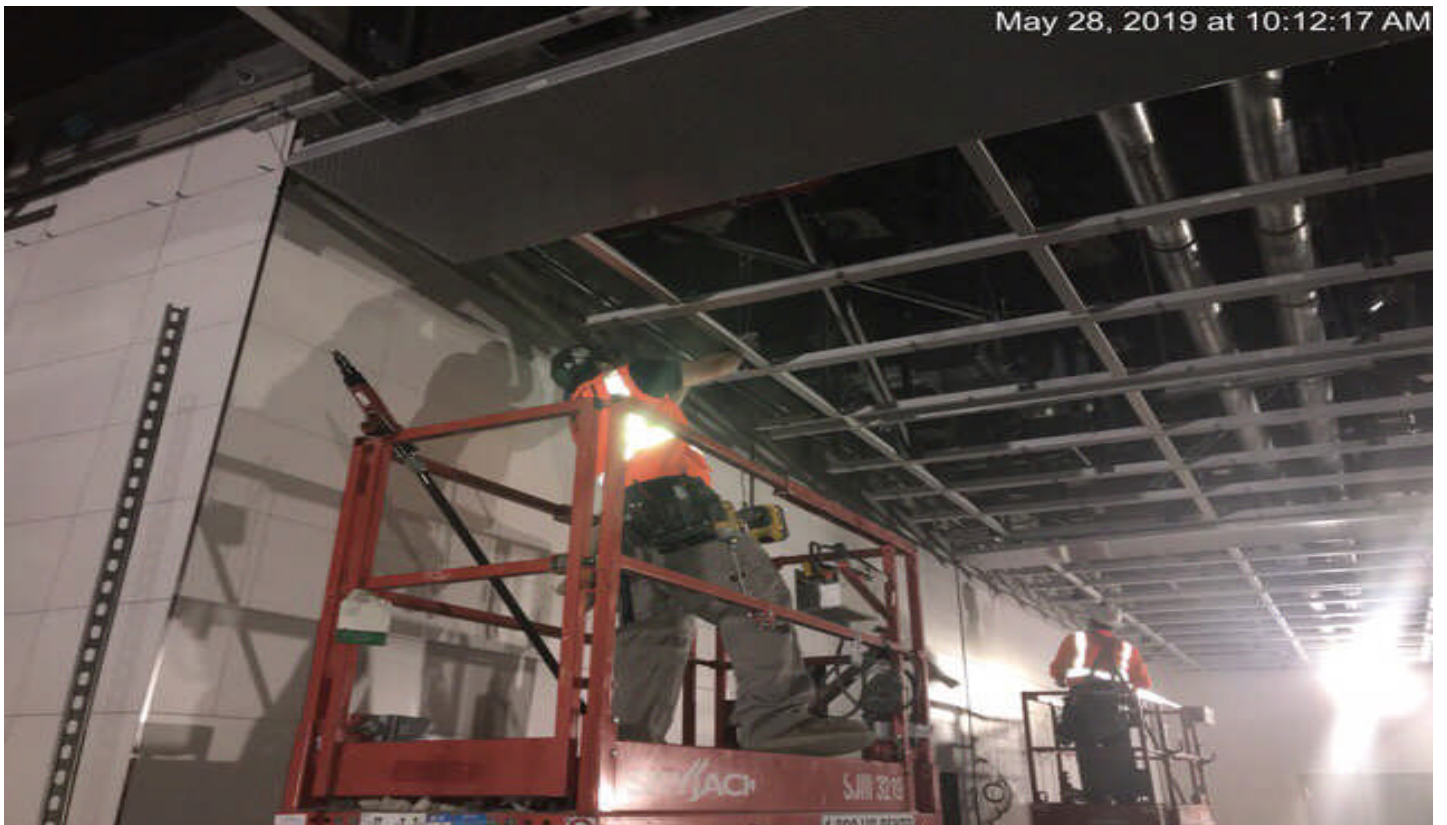
EXPOSITION/CRENSHAW STATION – Installation of the metal ceiling panel at the concourse level.
