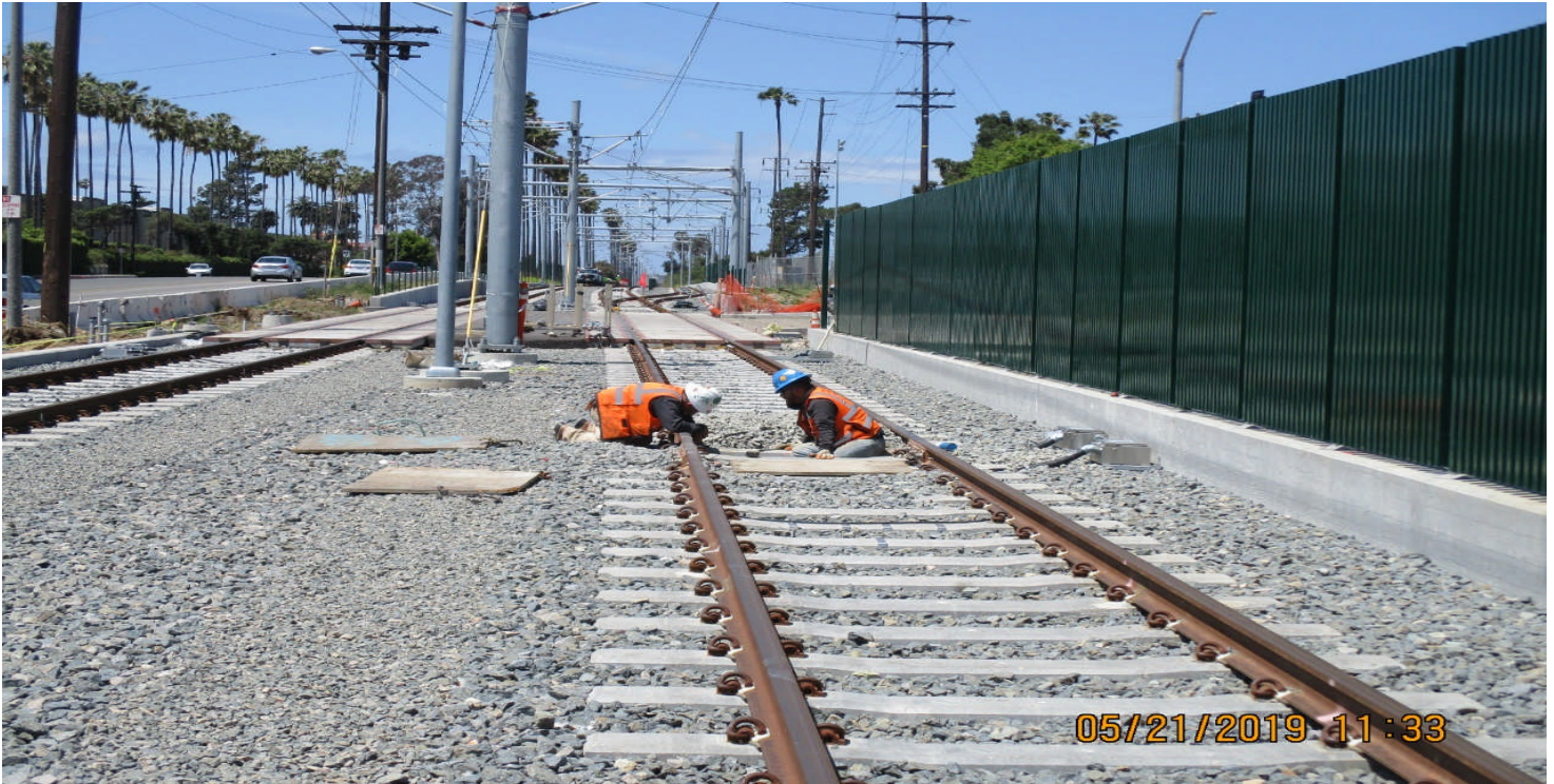
HIGH STREET- Guideway between High St. to West Station re-consolidation of track ballast rock.
