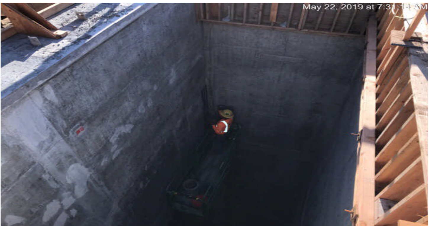
MARTIN LUTHER KING JR. STATION- Finish work for Elevator 1 & 2 at the concourse level.
