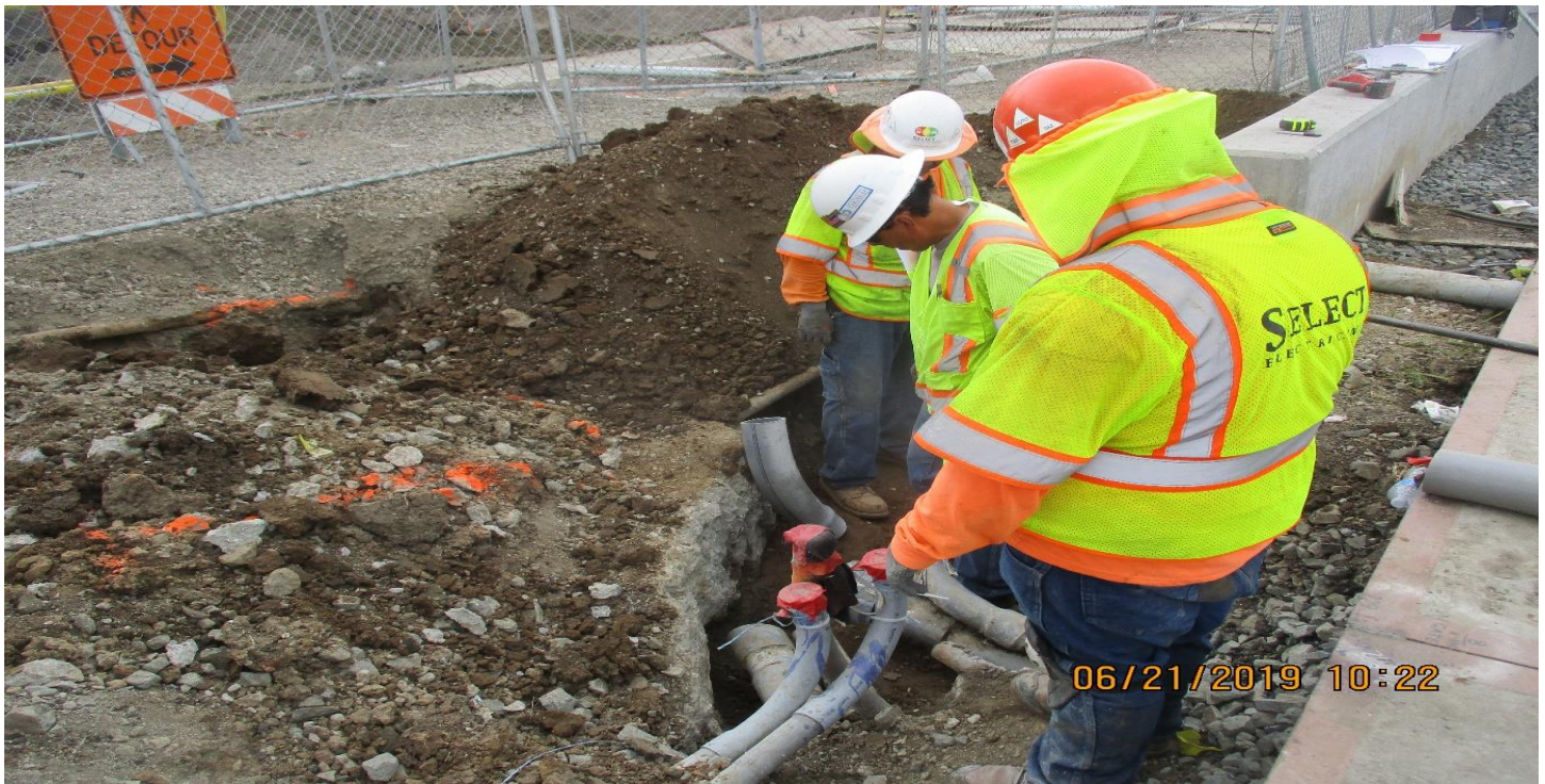
FLORENCE/CENTINELA - Select Electric Place conduits and pull boxes at Centinela and Florence crossing.
