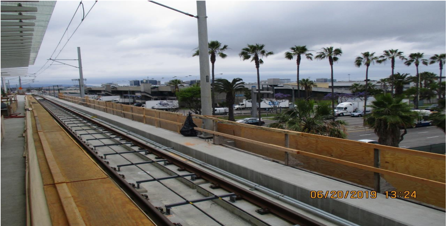
AVIATION/CENTURY- UP continue grout of North Bond track edge pavers and handrail at coping slab.
