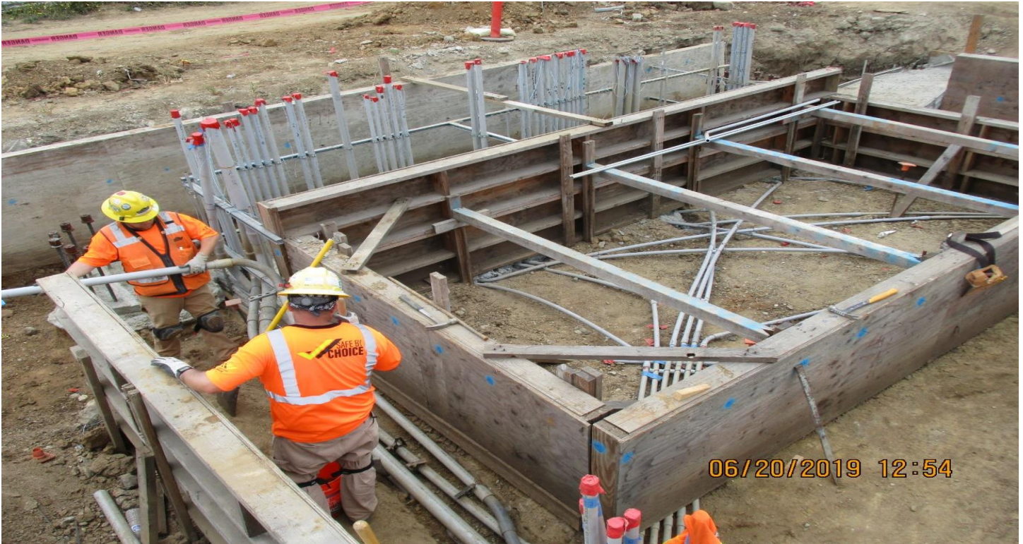
DOWNTOWN INGLEWOOD STATION- Guideway at Inglewood Station ticketing pavilion footing cleanout and grading.
