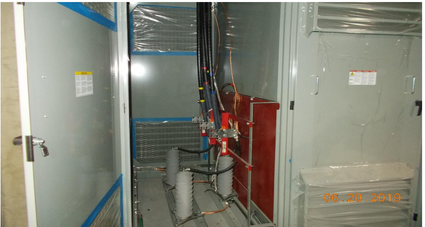
CRENSHAW/VERNON- PX1S high voltage terminations on cables.
