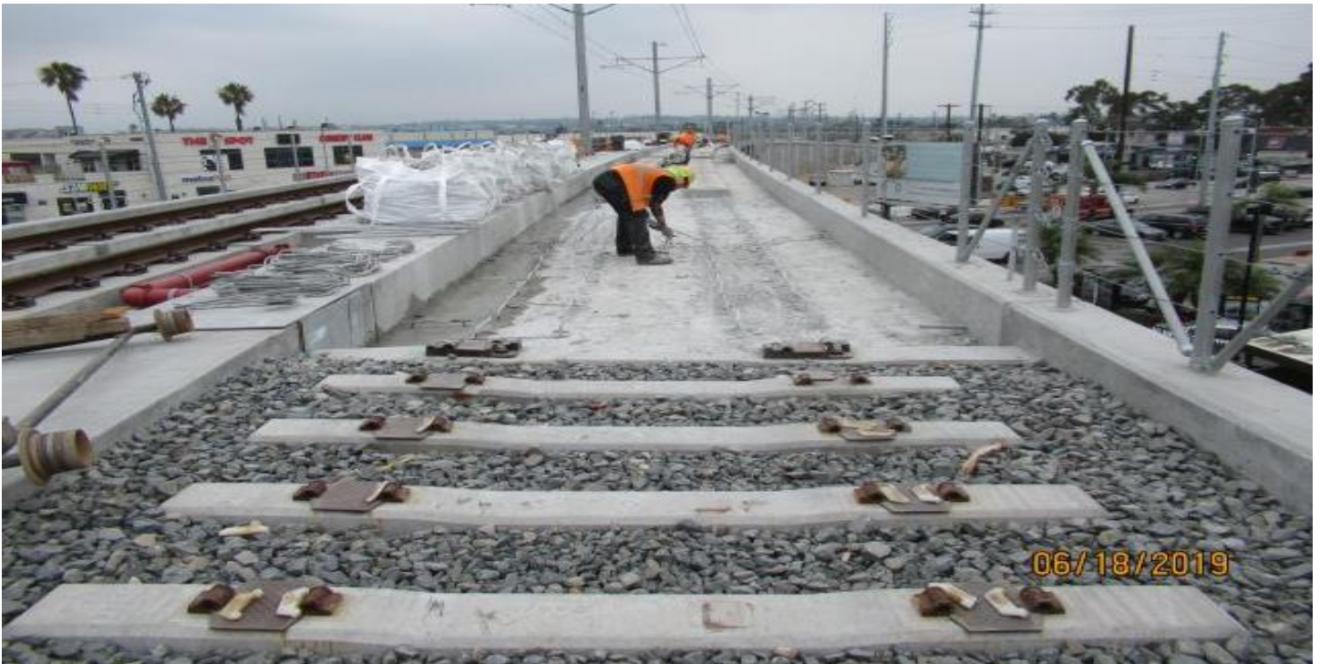
MANCHESTER BRIDGE- Manchester Bridge NB track WSCC removing existing rebar on demoed plinths.
