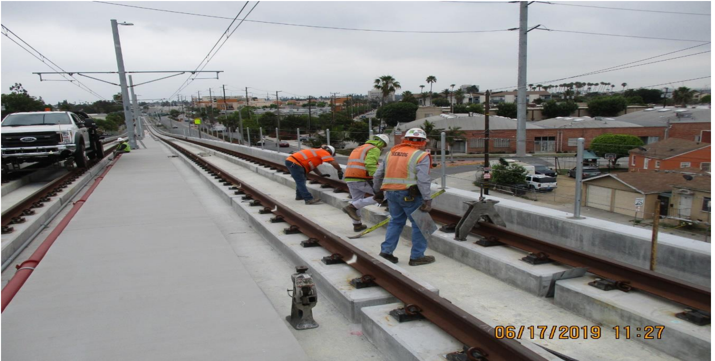
405 BRIDGE - CA Guideway at 405 UP line and shimming of NB track STA 149+00 to 154+00.
