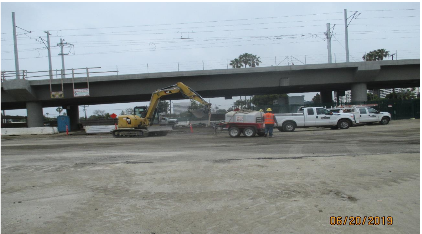
AVIATION/CENTURY- Moving equipment to continue AC demo at the Aviation Station yard.
