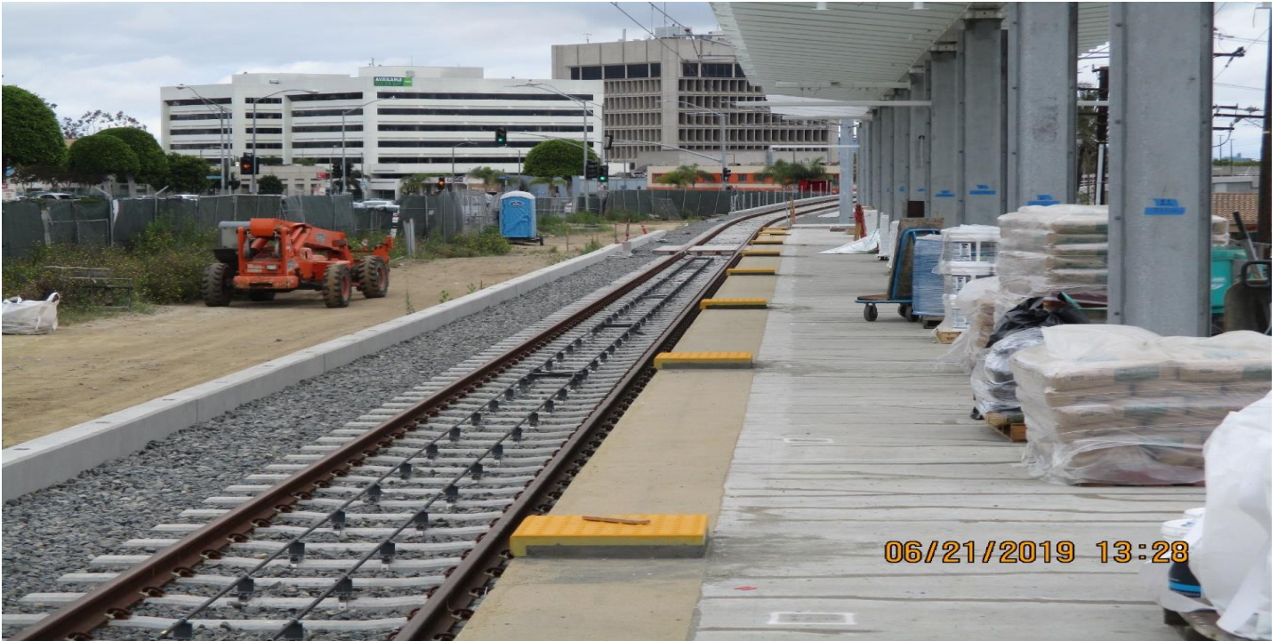
DOWNTOWN INGLEWOOD STATION- Guideway at Downtown Inglewood Station platform and ticketing pavilion overview.
