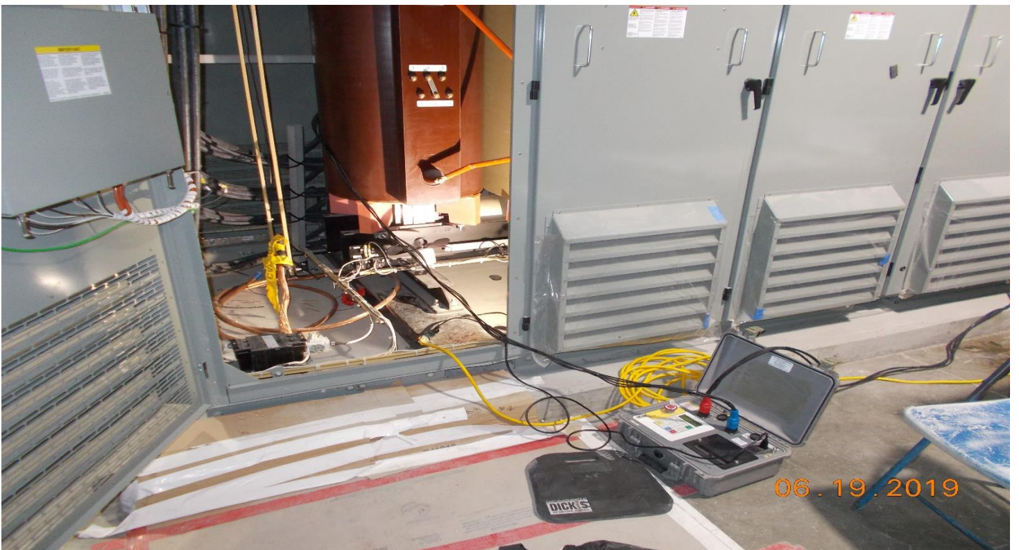
CRENSHAW/EXPO- Aux Power north PX2N testing
