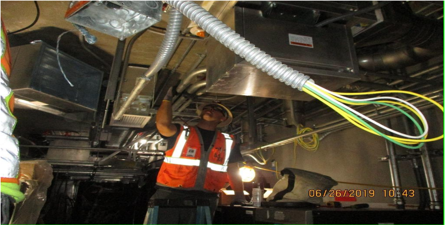
FLORENCE/HINDRY - WSCC Electric Westchester Veteran Station running Intrusion and Fire Alarm Conduit in the TC&C room.
