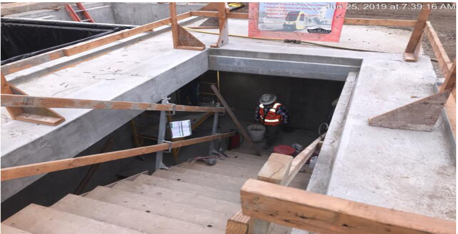
MARTIN LUTHER KING JR. STATION- Continued finish work from invert to concourse level at Emergency Exit #2.
