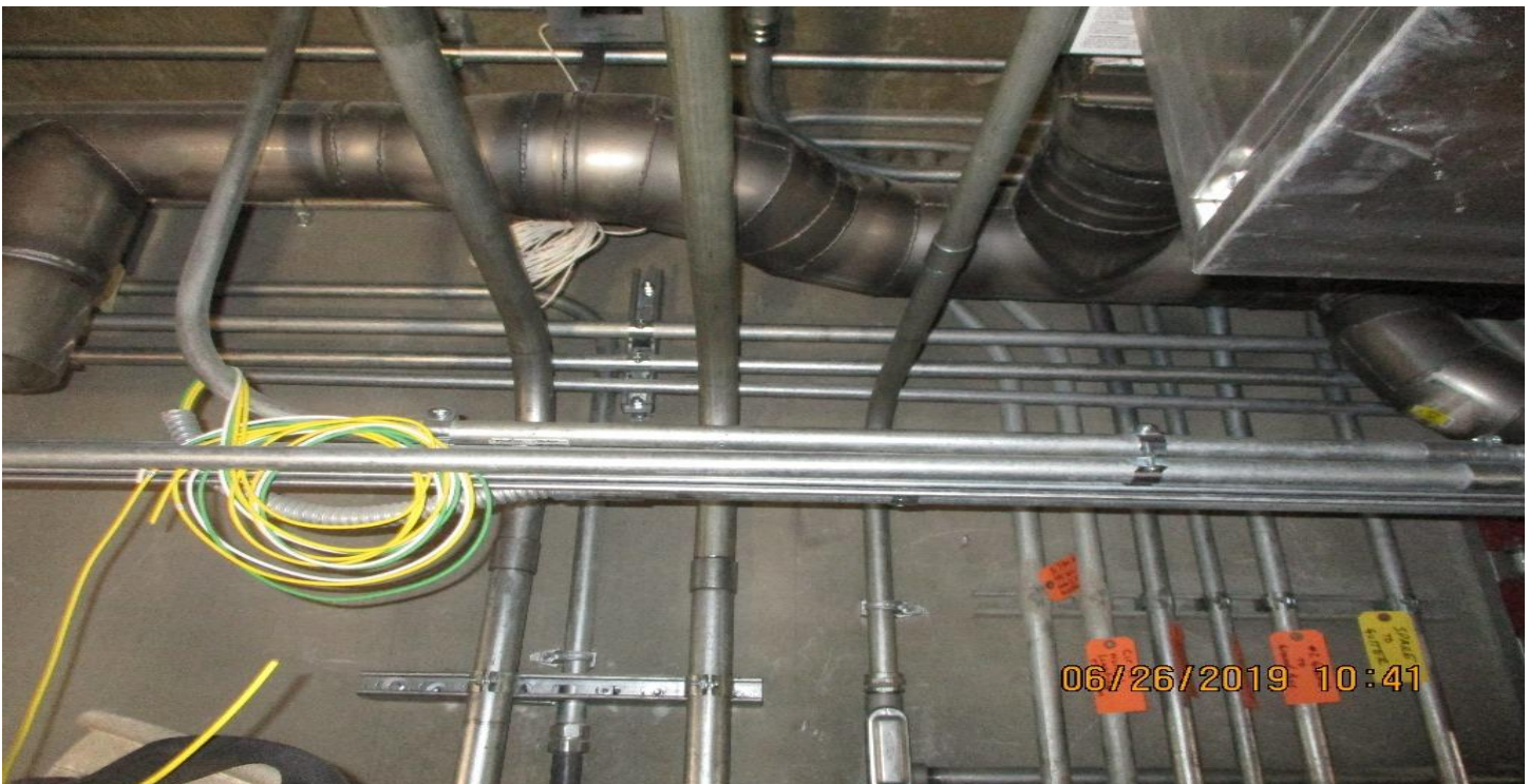
FLORENCE/HINDRY - WSCC Electric Westchester Veteran Station running Intrusion and Fire Alarm Conduit in the TC&C room
