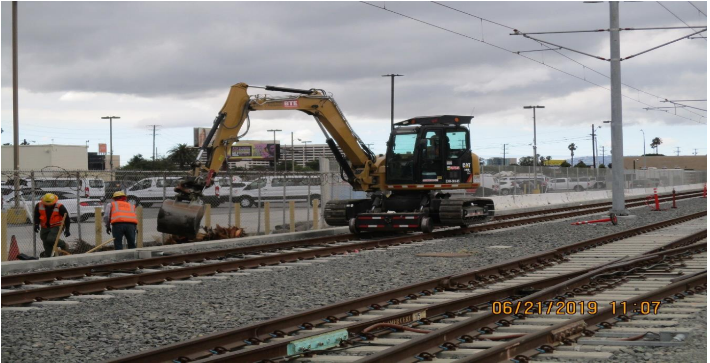
GUIDEWAY-ARBOR VITAE- A Guideway north Arbor Vitae clearing and grubbing and prep for drainage swale.
