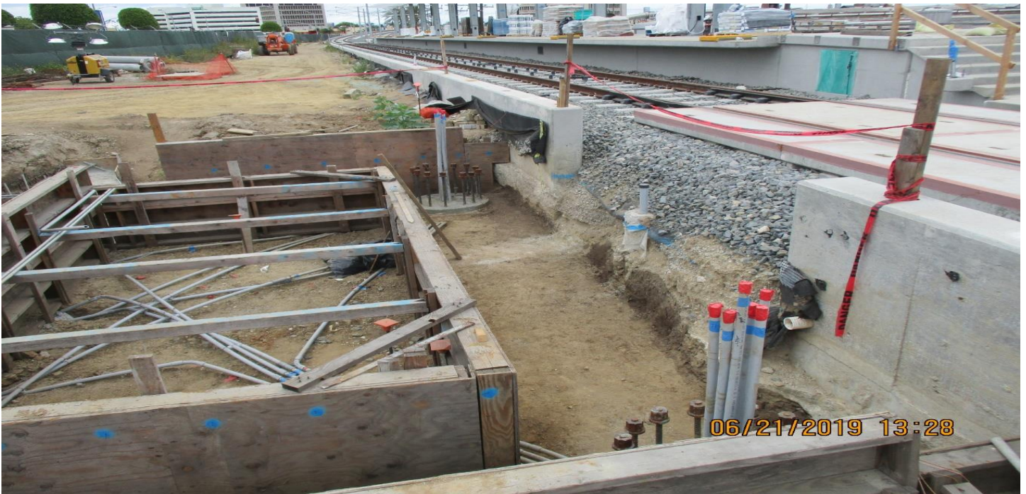
DOWNTOWN INGLEWOOD STATION- B1 Guideway at Downtown Inglewood Station platform and ticketing pavilion overview.
