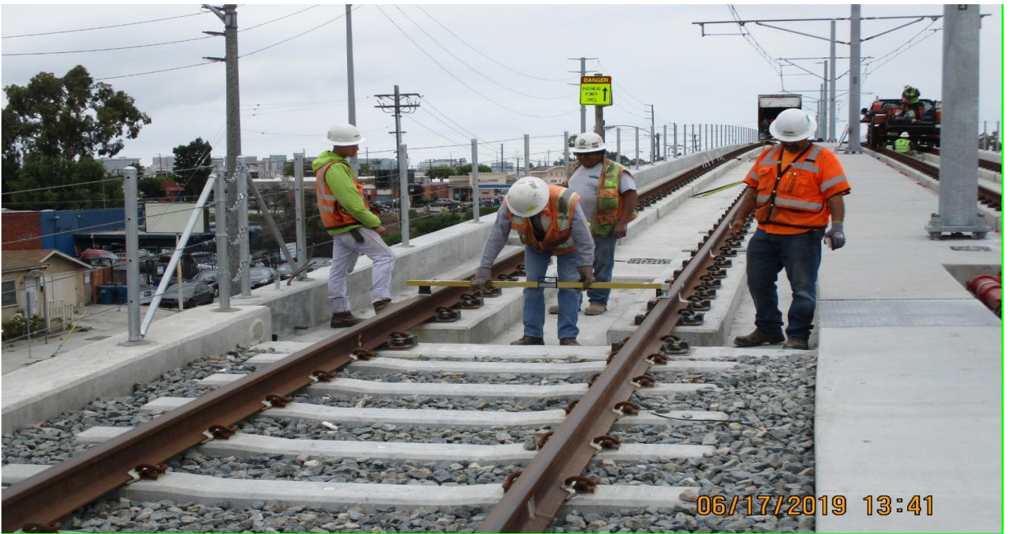
405 BRIDGE - A Guideway at 405 UP line and shimming of NB track STA 149+00 to 154+00.
