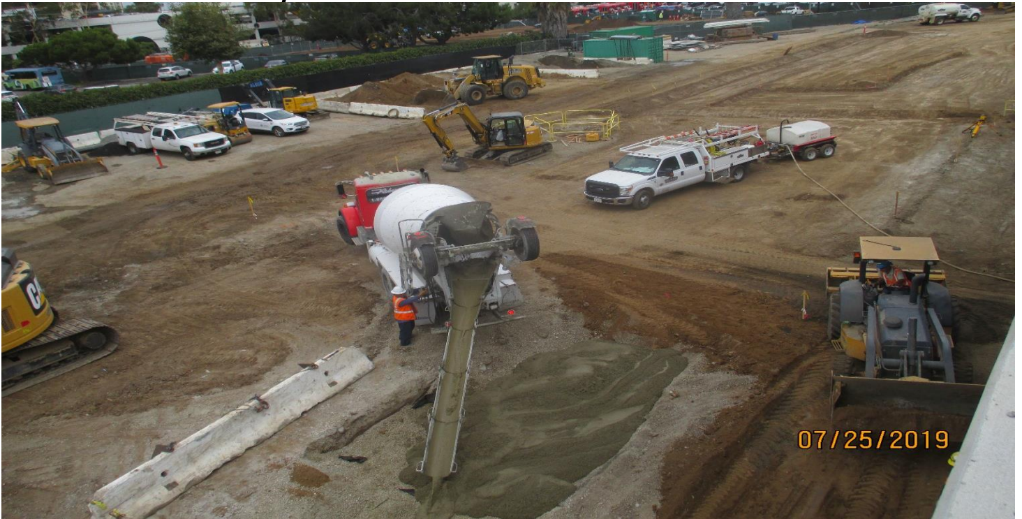
AVIATION/CENTURY- Slurry backfill of the interceptor pit at the Aviation Station yard.
