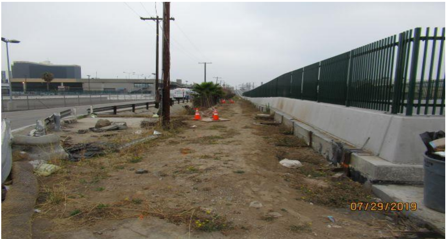
UG-1- 104th street north side no changes for UG1 Jet Fan conduit install.
