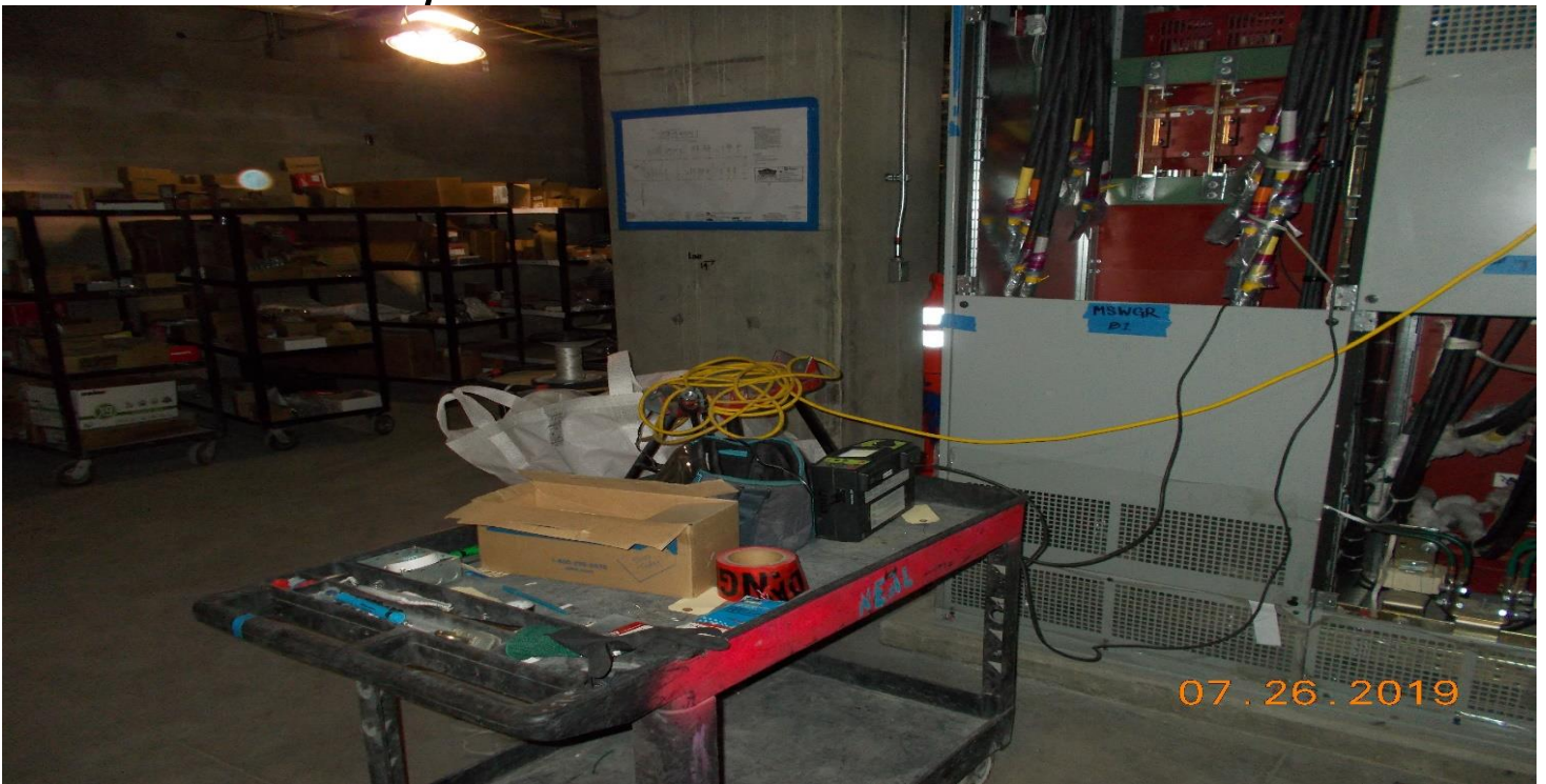
CRENSHAW/VERNON- NETE performing megger testing on MSWGR-N.
