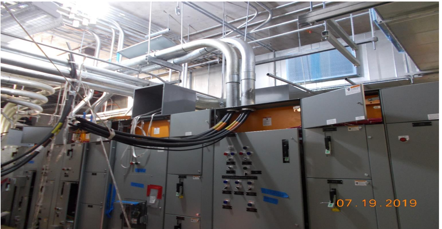
EXPOSITION/CRENSHAW STATION – Aux Power north MCC1N emergency fan cable feeds.
