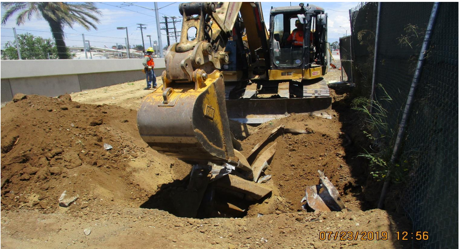
FLORENCE/LA BREA - WSCC Remove metal guard rail wall at WB Florence and La Brea.
