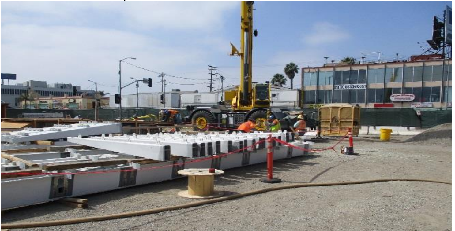
LEIMERT PARK STATION- Prep connection points for entrance canopy and Elevator 1 & 2 steel at the topside.
