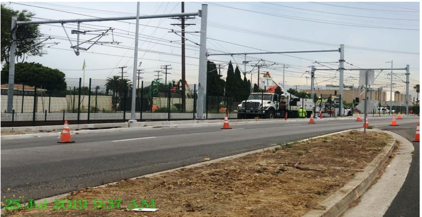
UG4- LKC installation of cantilever arm brackets for OCR Expo Station UG-4.
