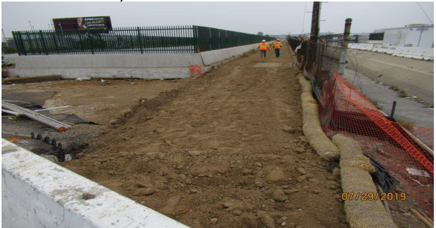
UG-1- 104th street south side no changes for UG1 Jet Fan conduit install.
