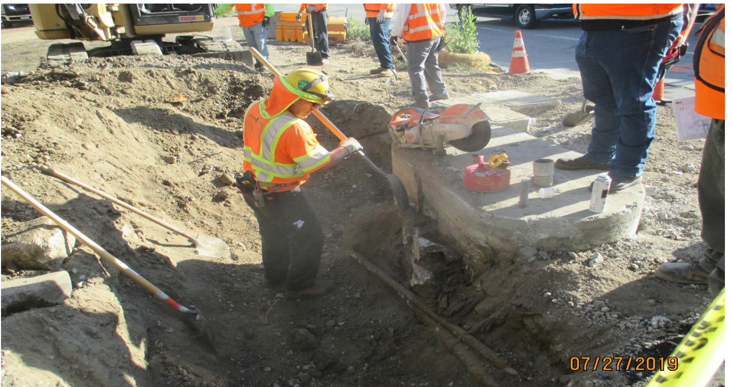
AVIATION/CENTURY- Existing foundation to be removed at the NW corner of Aviation.
