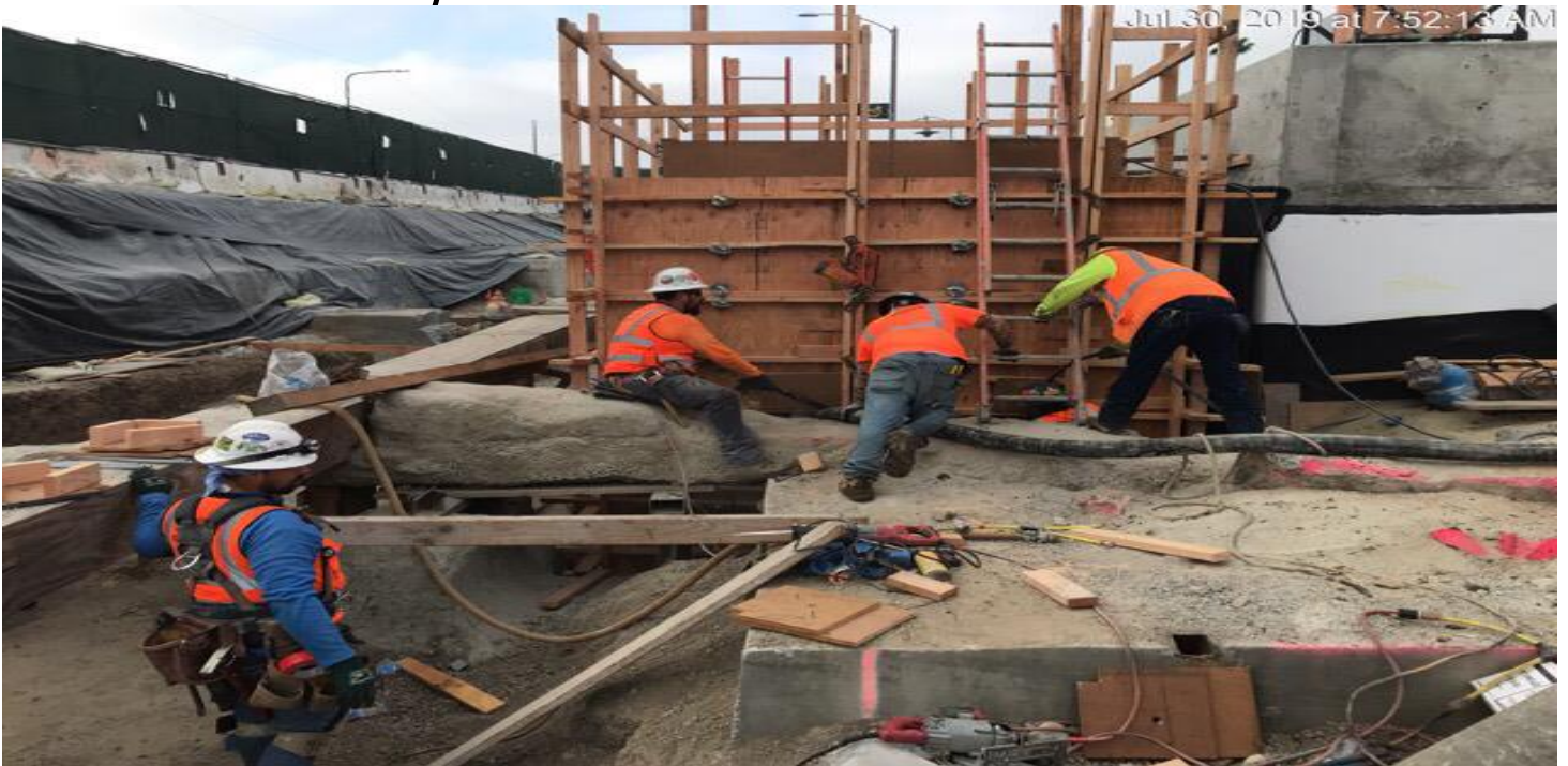
MARTIN LUTHER KING JR. STATION- Continued installation of water line vault at the topside.
