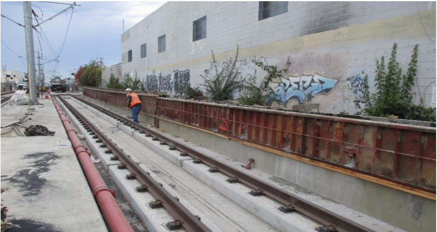
UG3- Continued installation of barrier wall along the track of the southbound portal.
