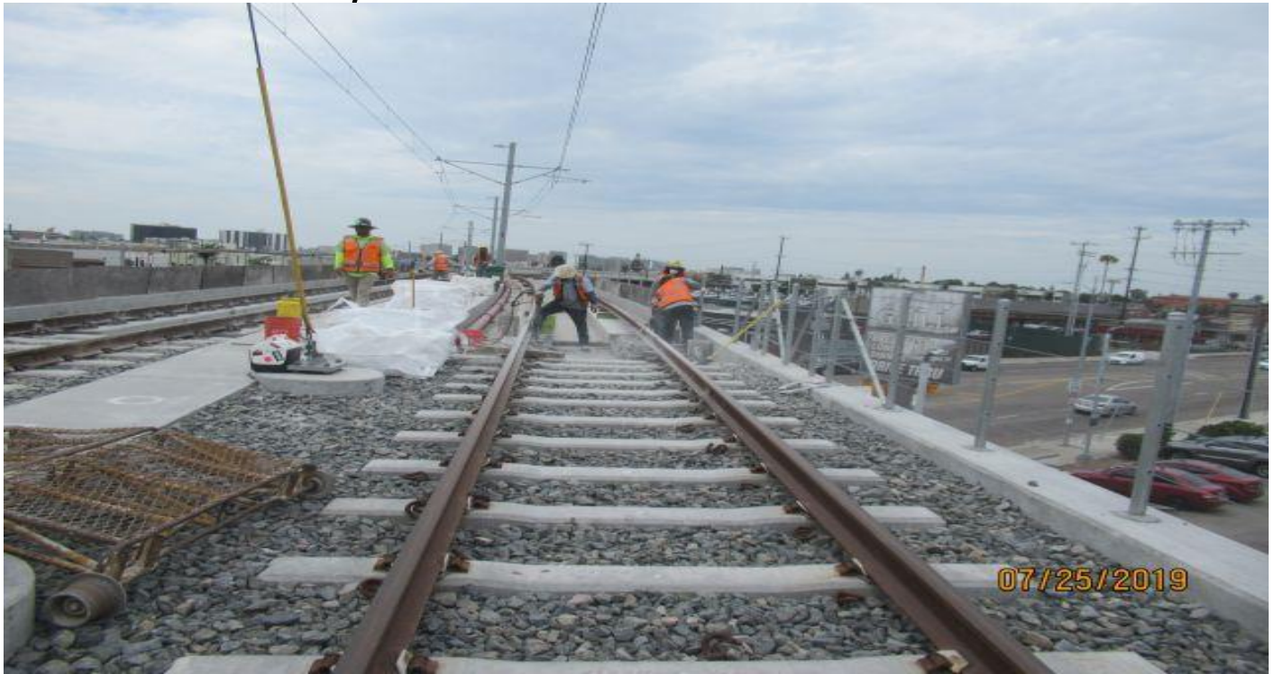
MANCHESTER BRIDGE- WSCC concrete crew demoing out required plinths on SB track.
