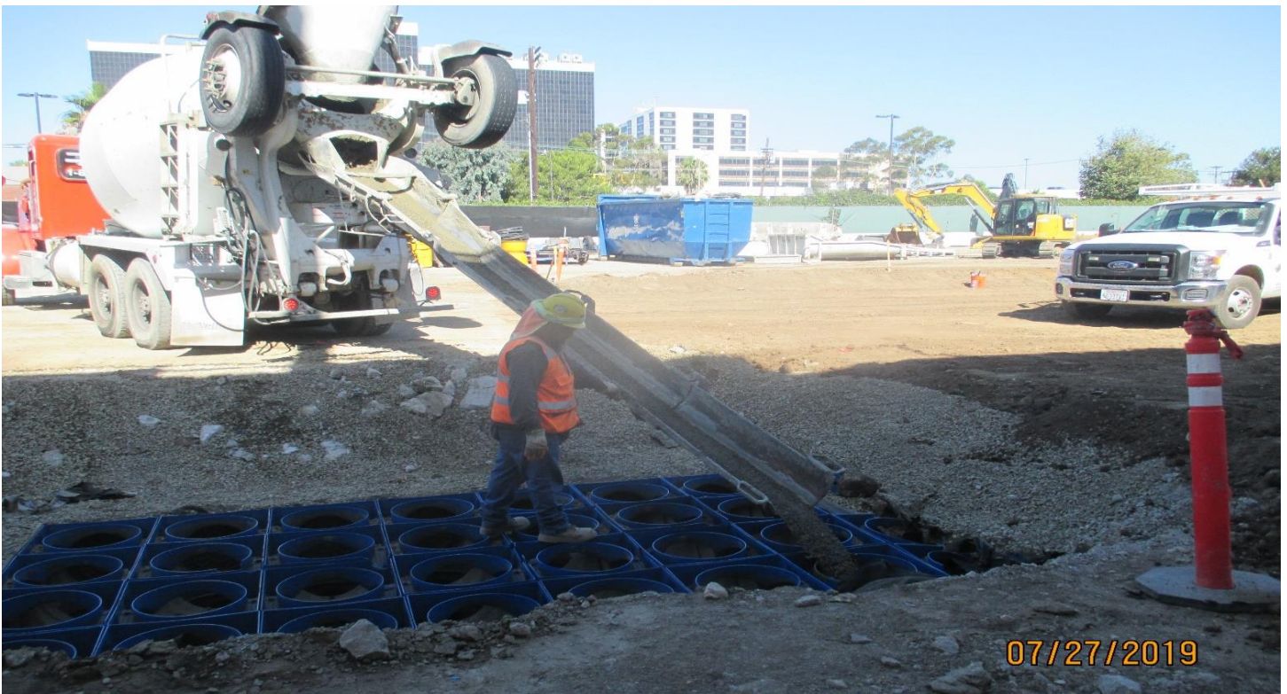
AVIATION/CENTURY- Slurry backfill of the interceptor pits at the Aviation Station yard.
