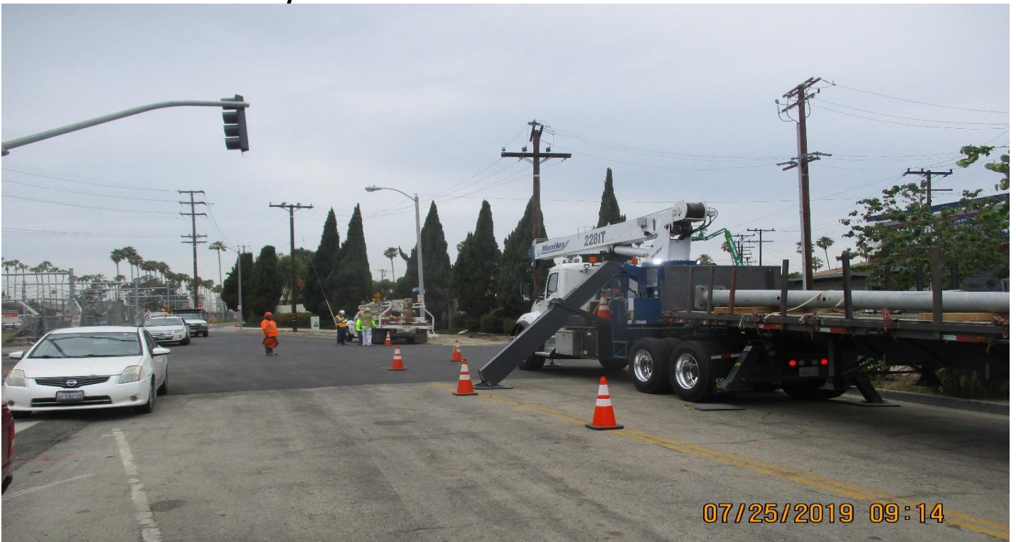
HIGH STREET- Select Electric Stand TS and SL poles at High and Redondo.
