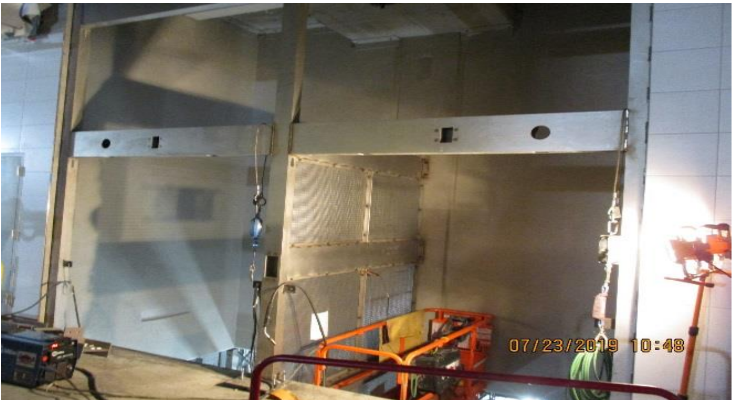
LEIMERT PARK STATION- Continued installation of elevator frame 3 & 4 at the platform level
