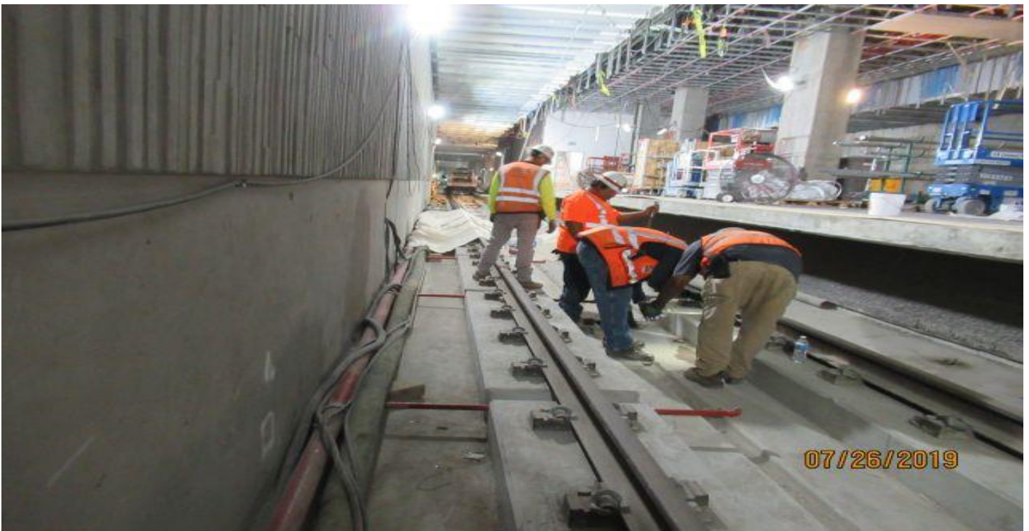
EXPOSITION/CRENSHAW STATION – HCC adjusting alignment on NB track at Expo. station platform.
