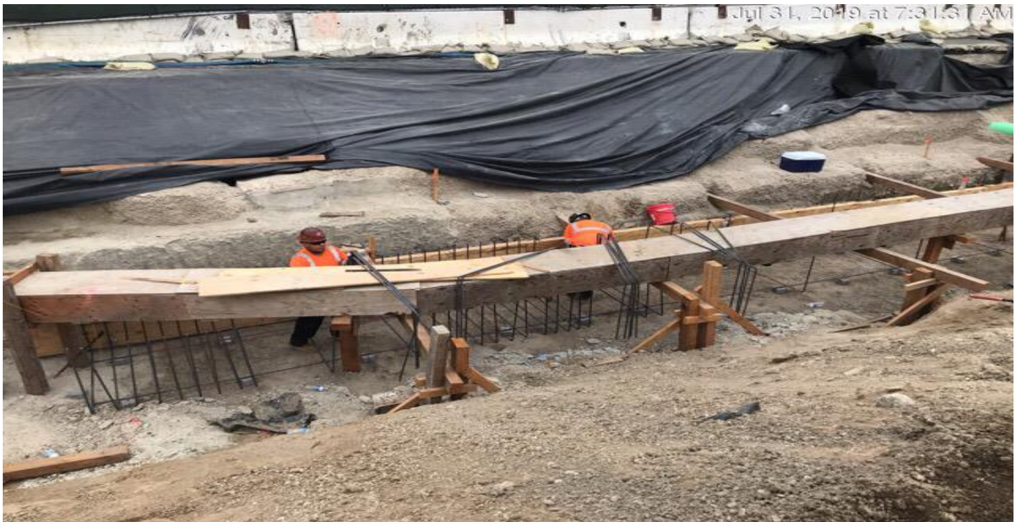
MARTIN LUTHER KING JR. STATION- Installation of rebar for C Line encasement at the topside.
