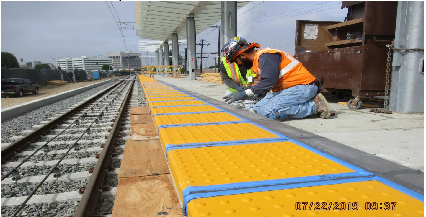
FLORENCE/LA BREA - Carrara Marble Place grout in yellow paver joints at La Brea Sta.
