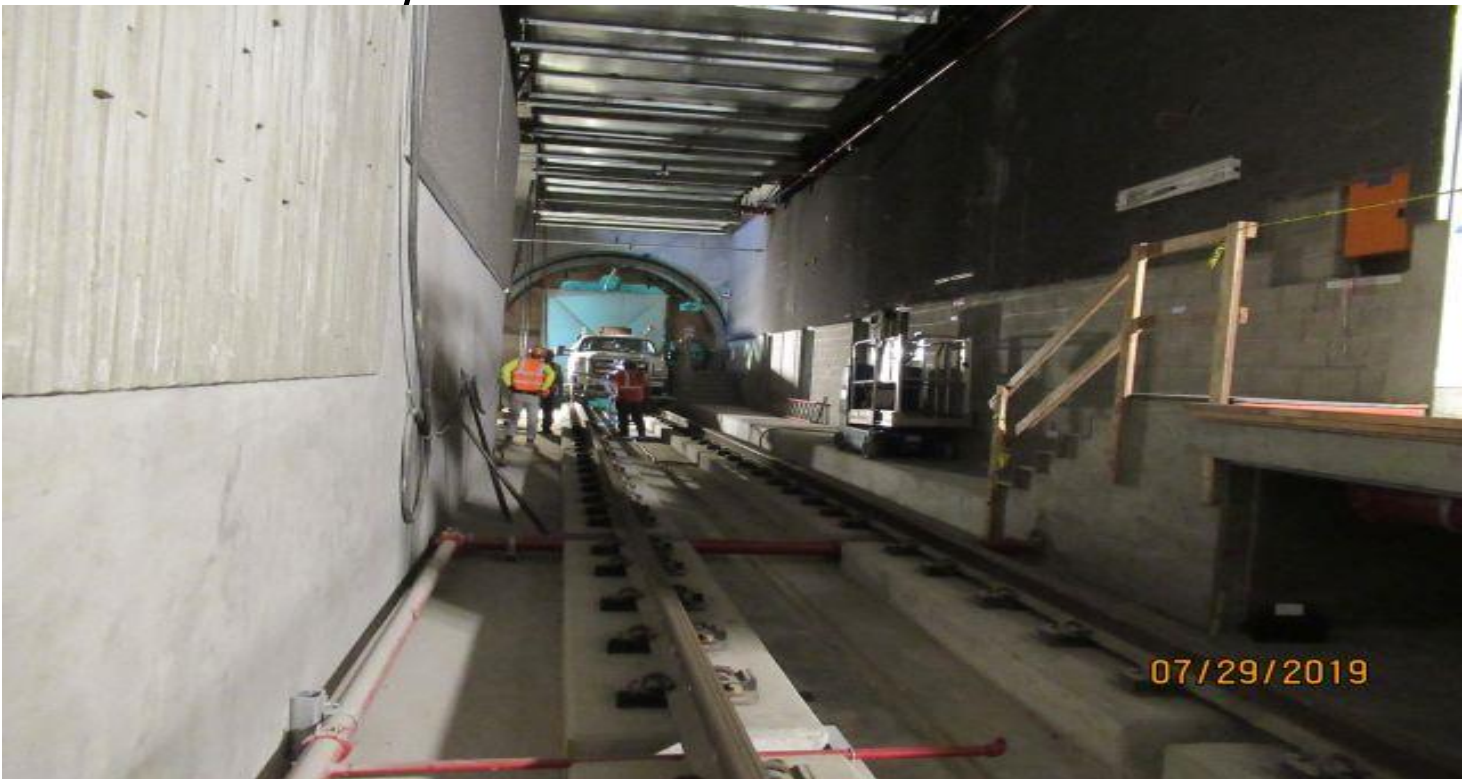
UG4- HCC on SB track in UG4 at MLK platform station.
