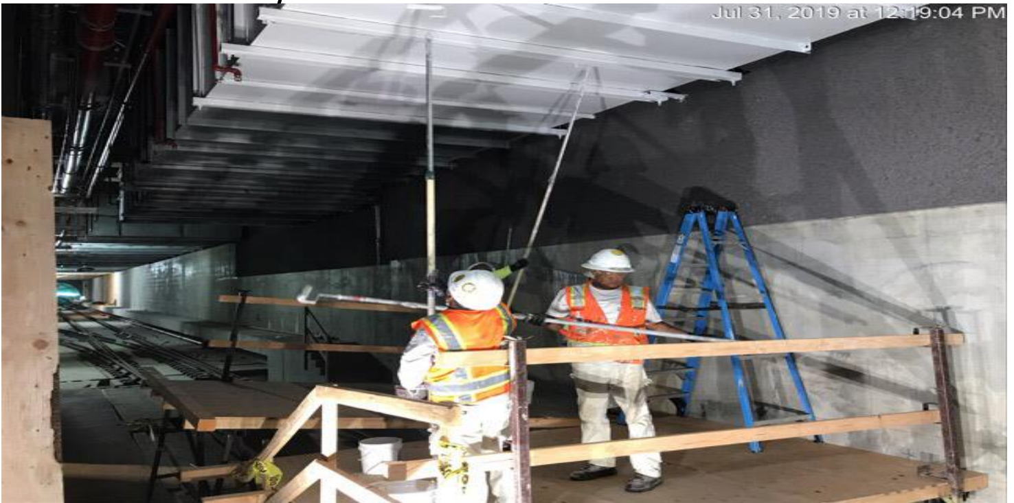
EXPOSITION/CRENSHAW STATION – Painting on southbound OTE vent duct at the invert level.
