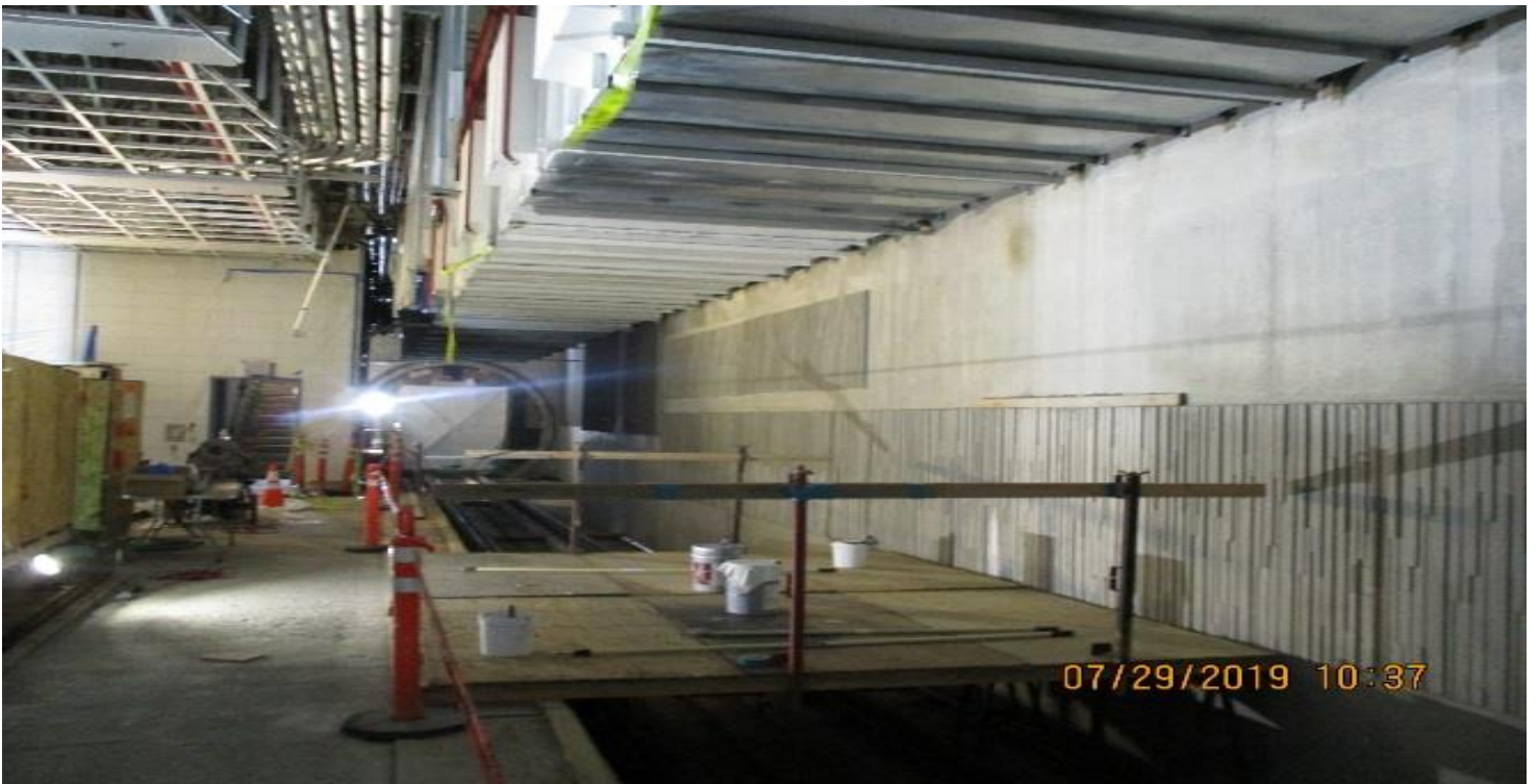
LEIMERT PARK STATION- Painting on northbound OTE vent duct at the invert level.
