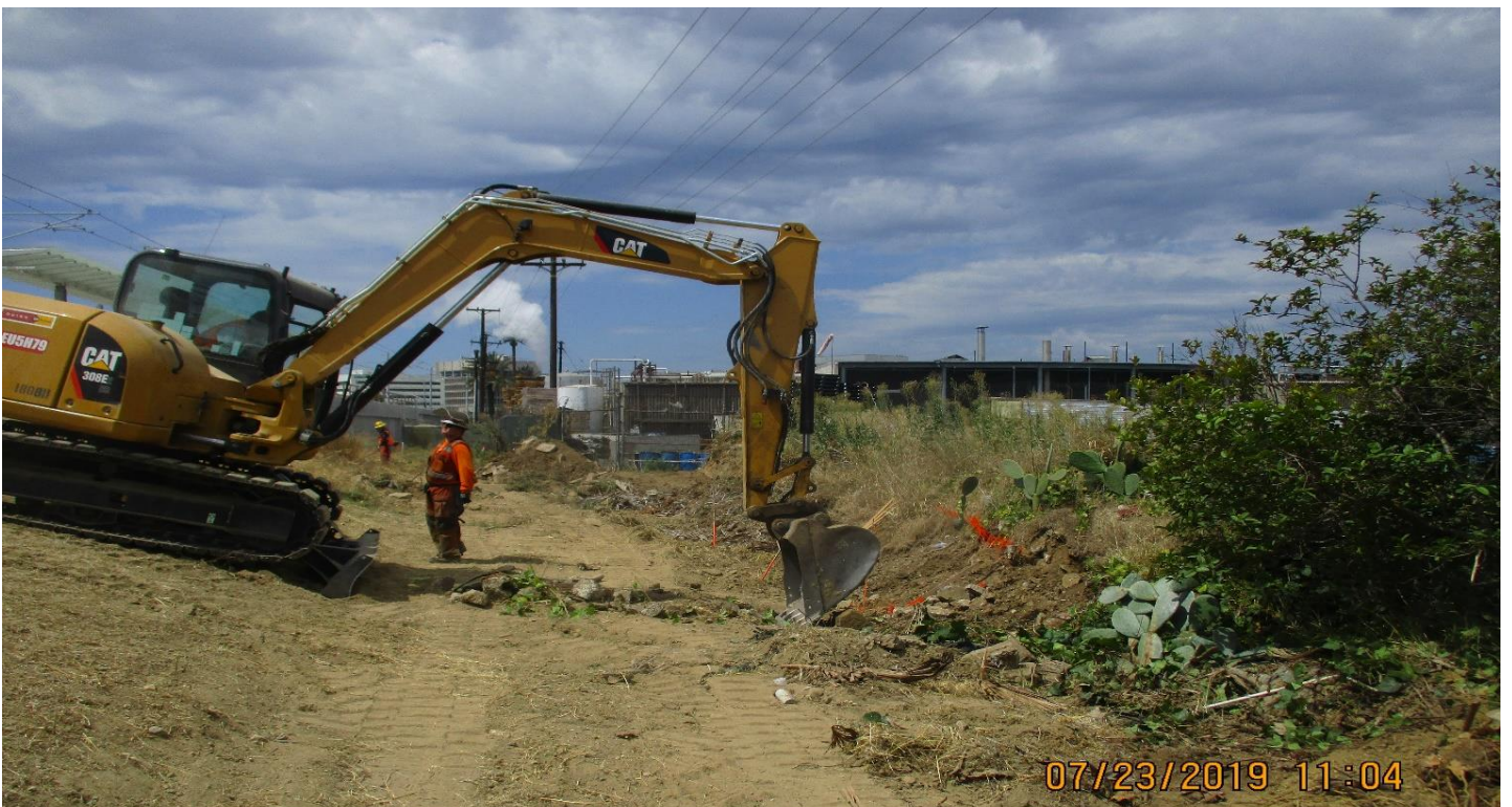
FLORENCE/LA BREA- WSCC Making grade and clear and grub for fence on north side of La Brea Sta.
