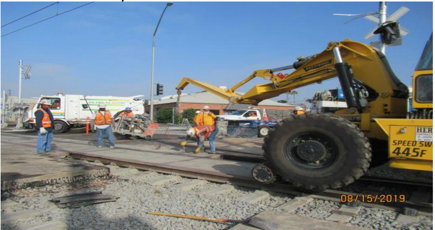
FLORENCE/HINDRY - HCC Speed Swing removing field crossing panels on SB track at Hindry grade crossing.
