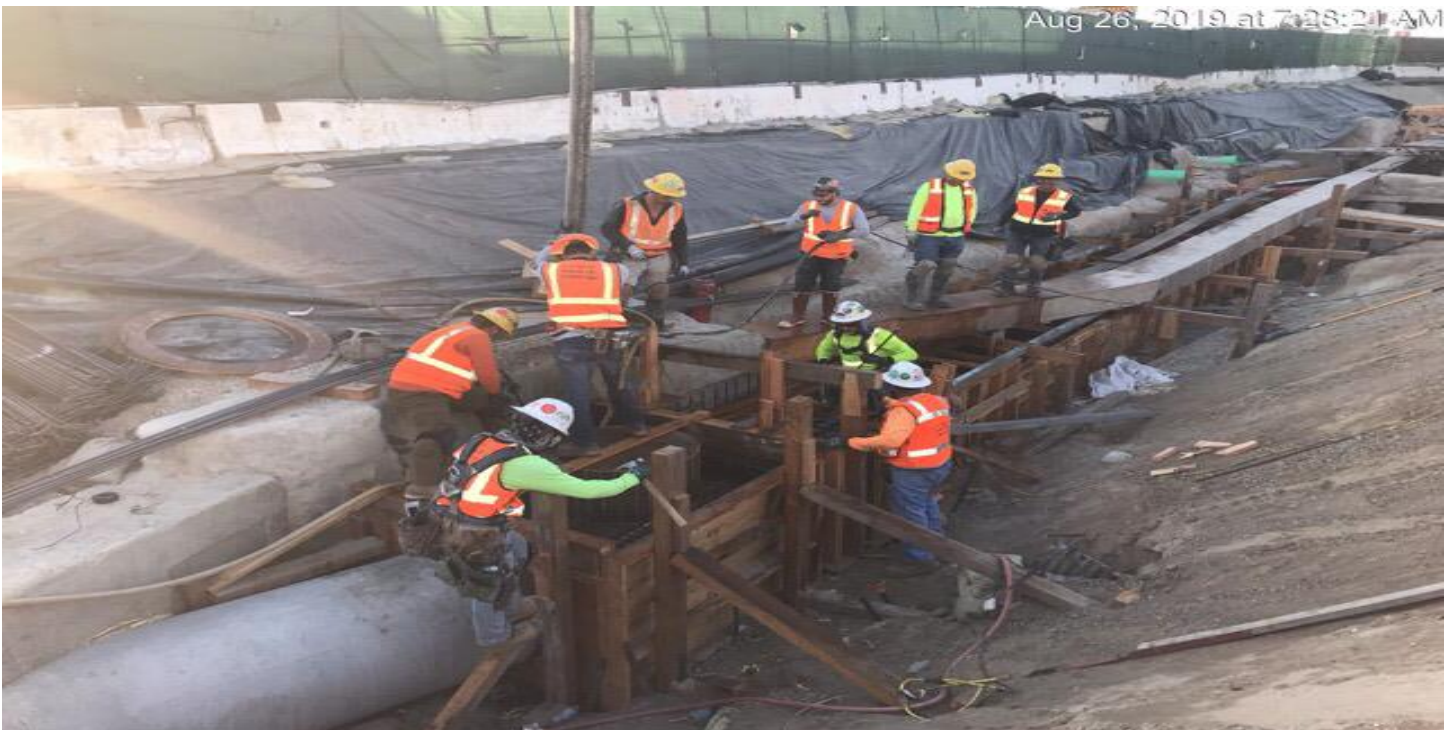
MARTIN LUTHER KING JR. STATION- Continued installation of wall forms for C Line encasement at the topside.
