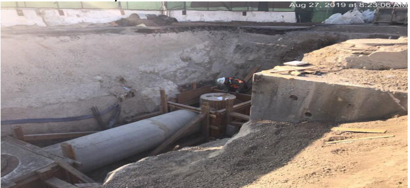
MARTIN LUTHER KING JR. STATION- Continued installation of wall forms for Manhole #19 at the topside.
