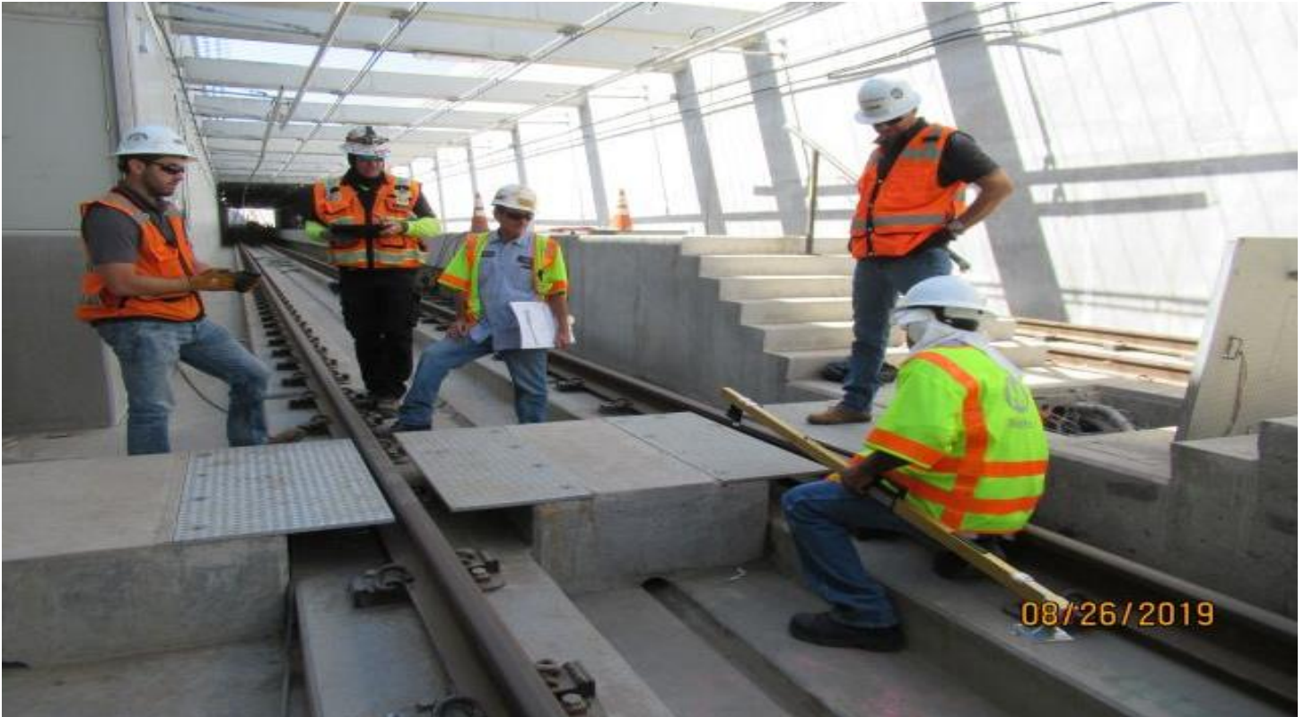
UG-1- Metro inspection walk in UG1 discussion of emergency walkway plate gaps on rails.
