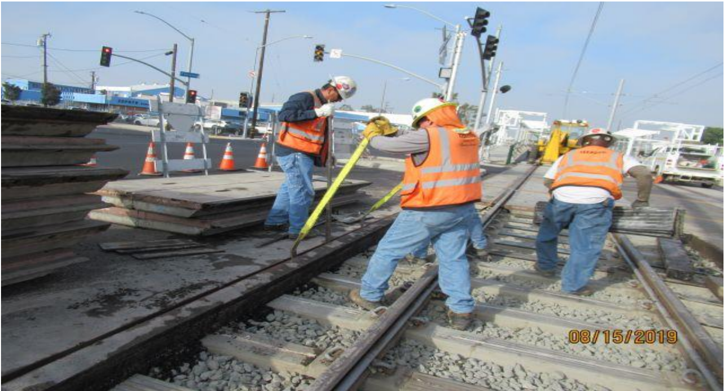
FLORENCE/HINDRY - HCC removing asphalt edge on NB track at Hindry grade crossing.
