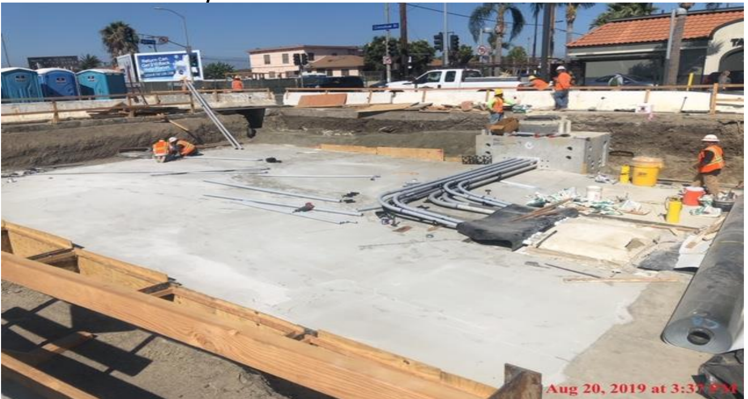
UG3- Continued installation of conduit on intersection of 60th and Crenshaw Blvd.
