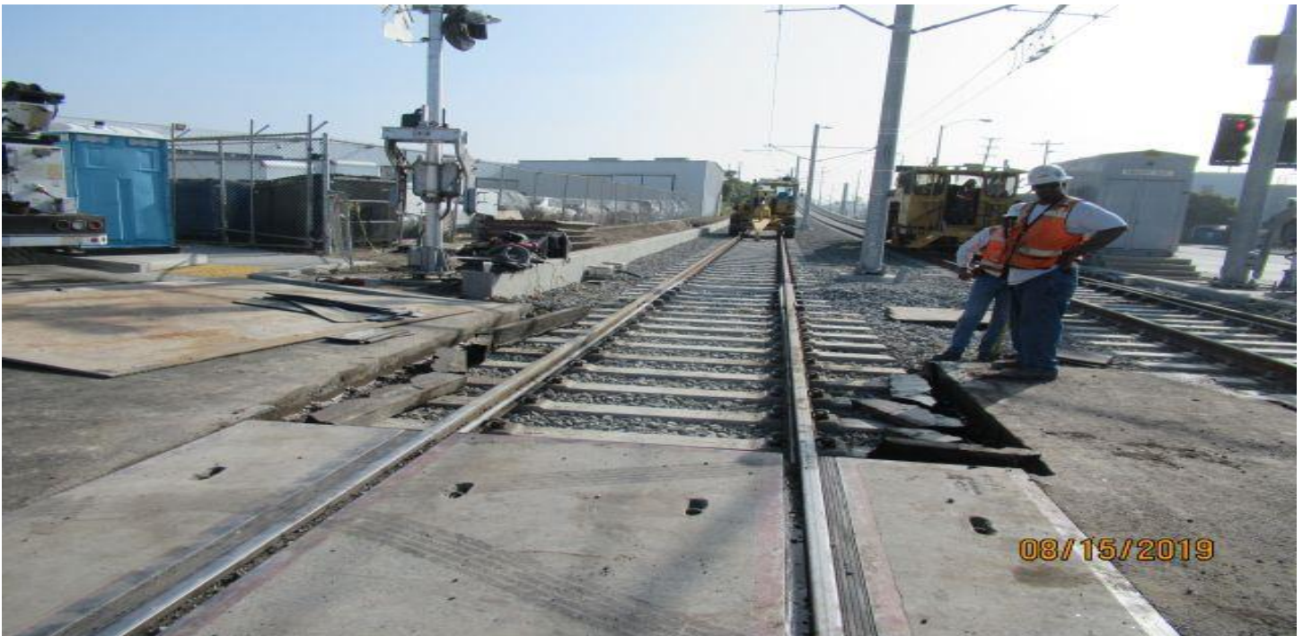
FLORENCE/HINDRY - SB track at Hindry grade crossing panels removed for re-tamping HCC.
