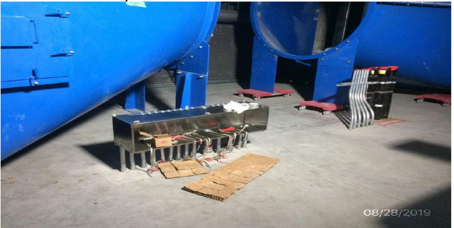
EXPOSITION/CRENSHAW STATION – Installation of gutter box for Emergency Ventilation Fan at the concourse level.
