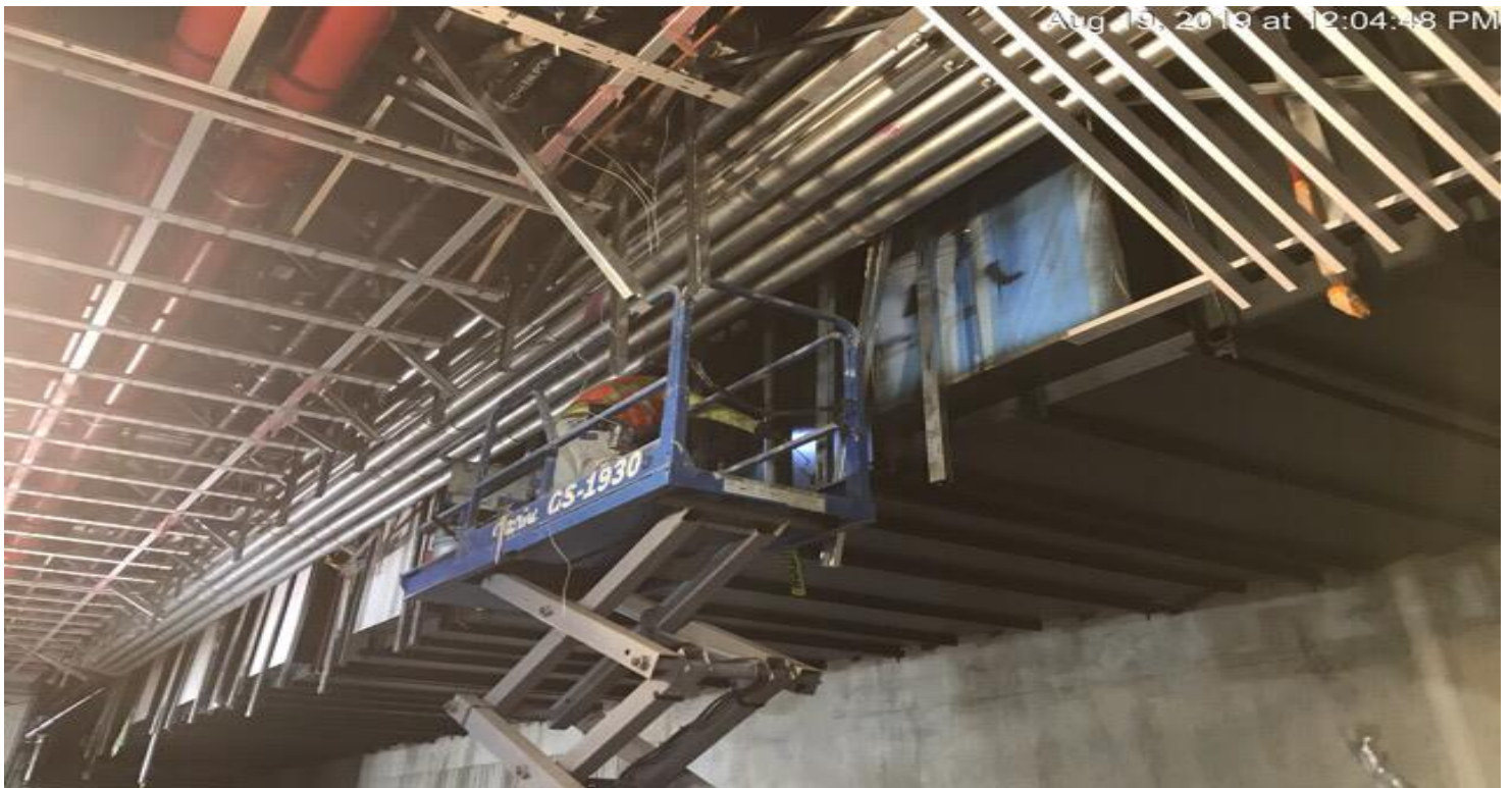
EXPOSITION/CRENSHAW STATION – Continued painting of southbound OTE vent duct at the invert level.
