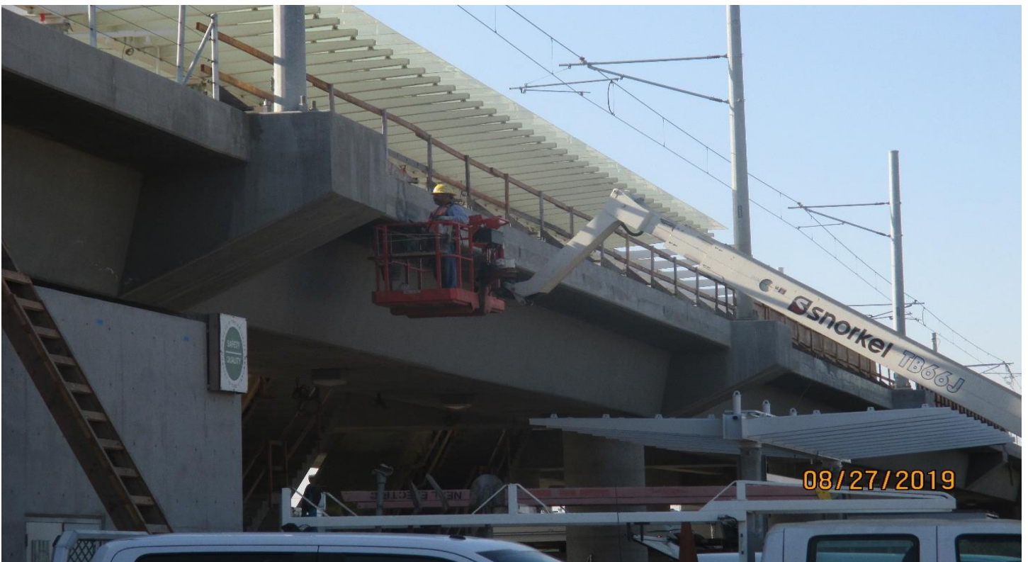
AVIATION/CENTURY- Class 1 concrete finish work for the Aviation Station bridge after the galvanized bolt replacement.
