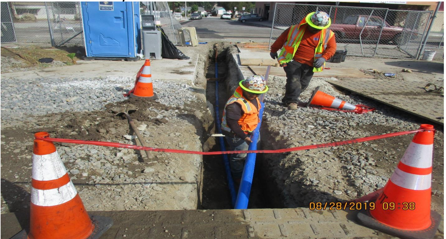
FLORENCE/WEST- Bali Const. Place 2" copper water line in West Sta parking lot.
