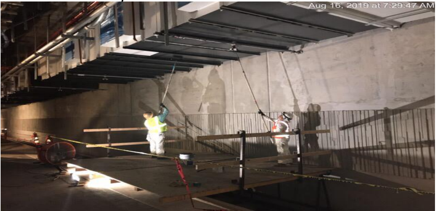
MARTIN LUTHER KING JR. STATION- Continued painting of southbound OTE vent duct at the invert level.
