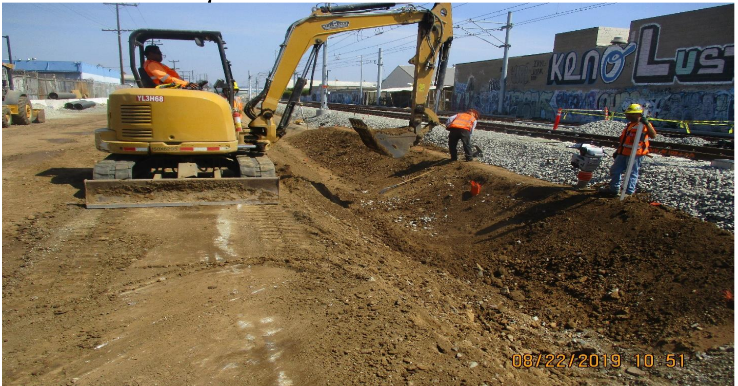
MANCHESTER BRIDGE- WSCC Grading for drainage swale at Portal area between arbor vitae & manchester bridge.
