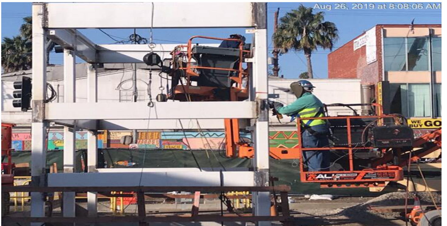
LEIMERT PARK STATION- Continued installation of entrance canopy steel for Elevator 1 & 2 at the topside.
