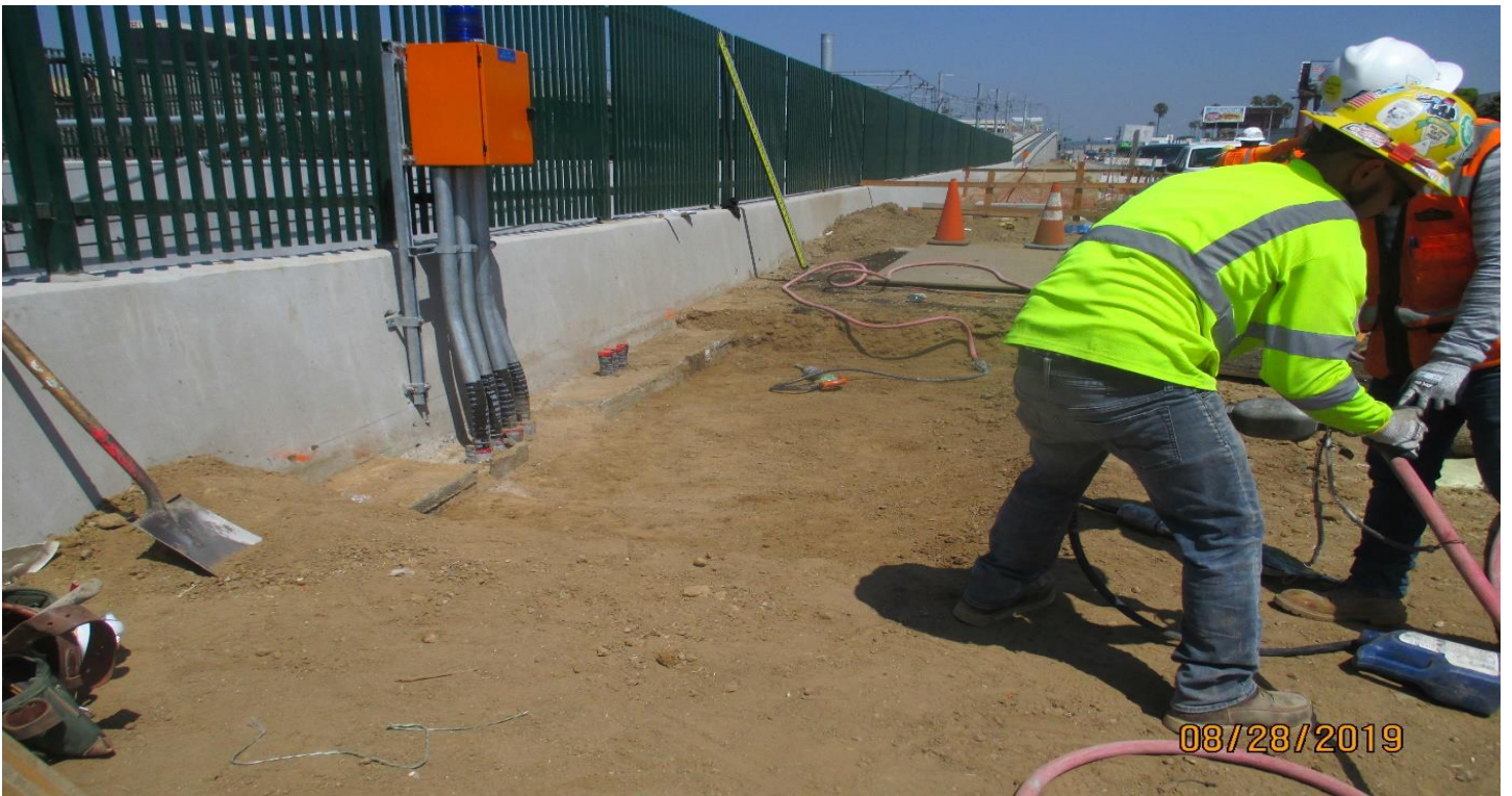
UG-1- Chipping the "U" wall concrete to build the BLS Trip Pad at UG-1.
