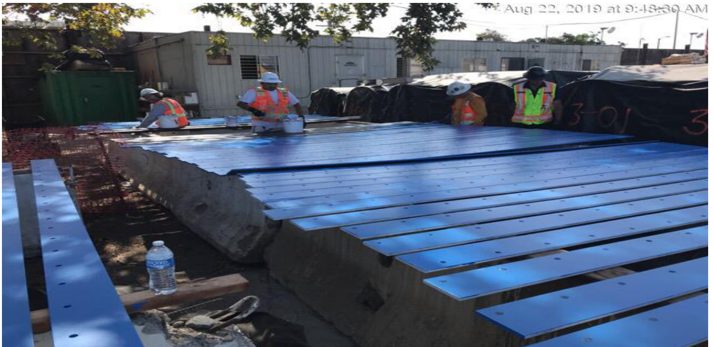
EXPOSITION/CRENSHAW STATION – Continued painting of connection plates for Emergency Ventilation Fans at the topside.
