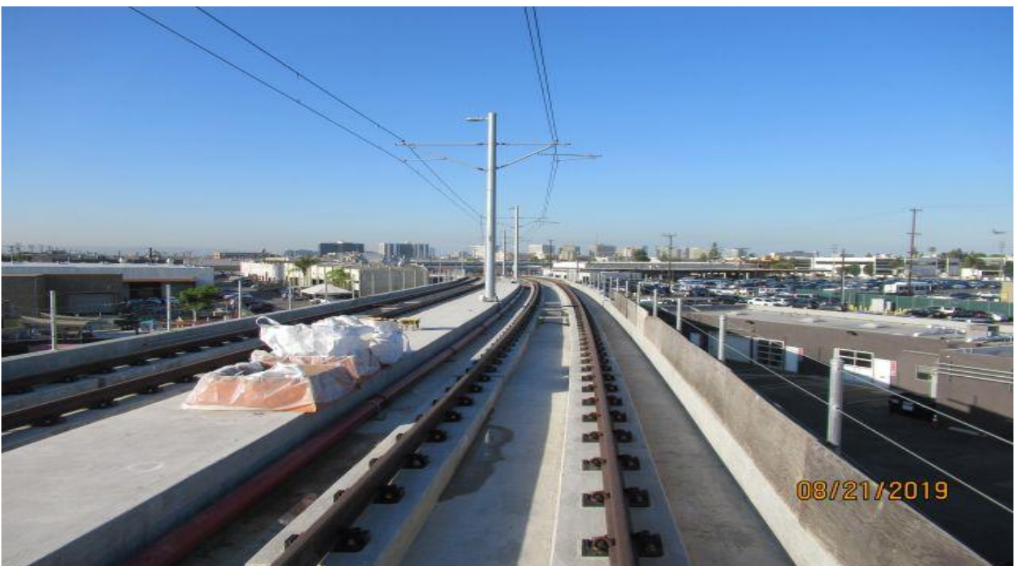
MANCHESTER BRIDGE- Manchester Bridge NB & SB tracks mid. point no construction being performed.
