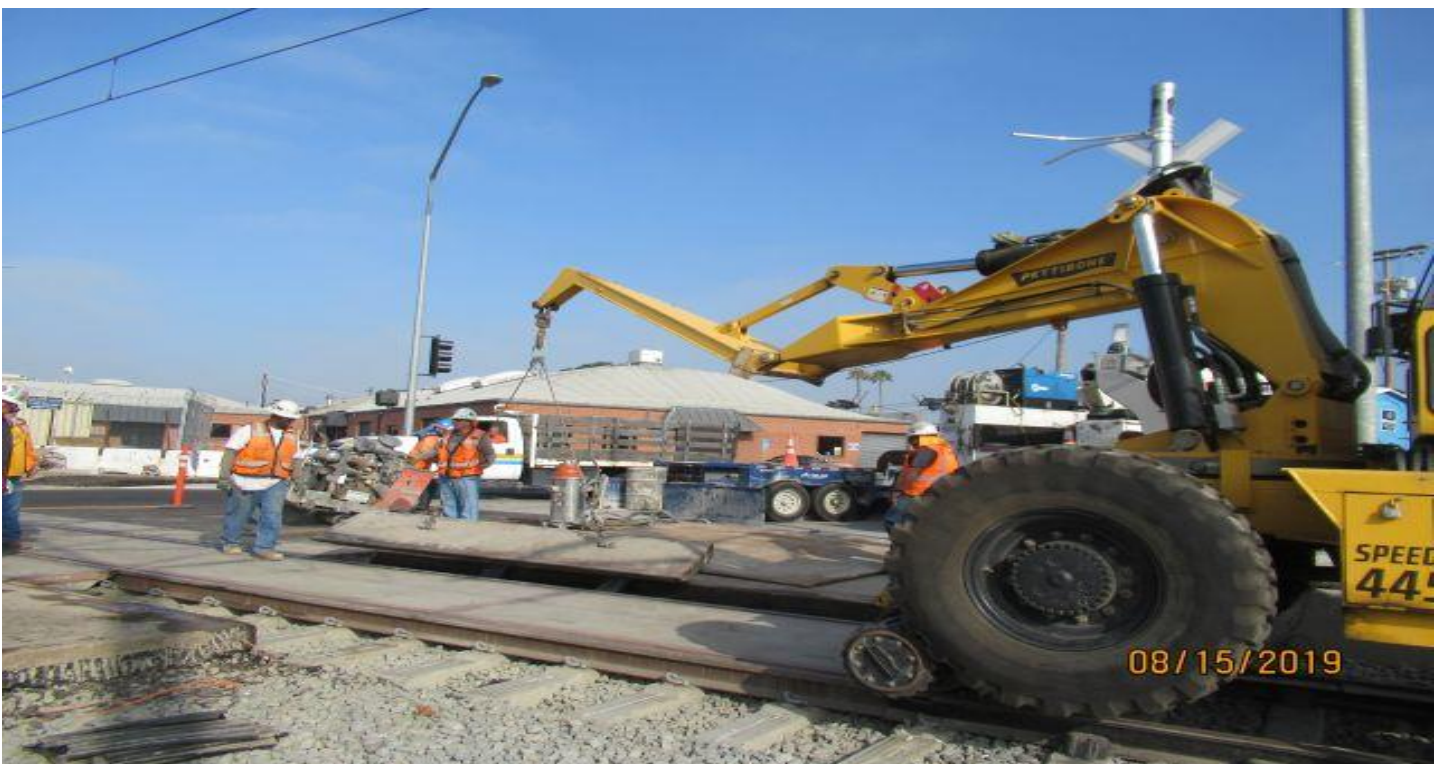
FLORENCE/HINDRY - HCC removing grade crossing panels on SB track to re-tamp at Hindry grade crossing.
