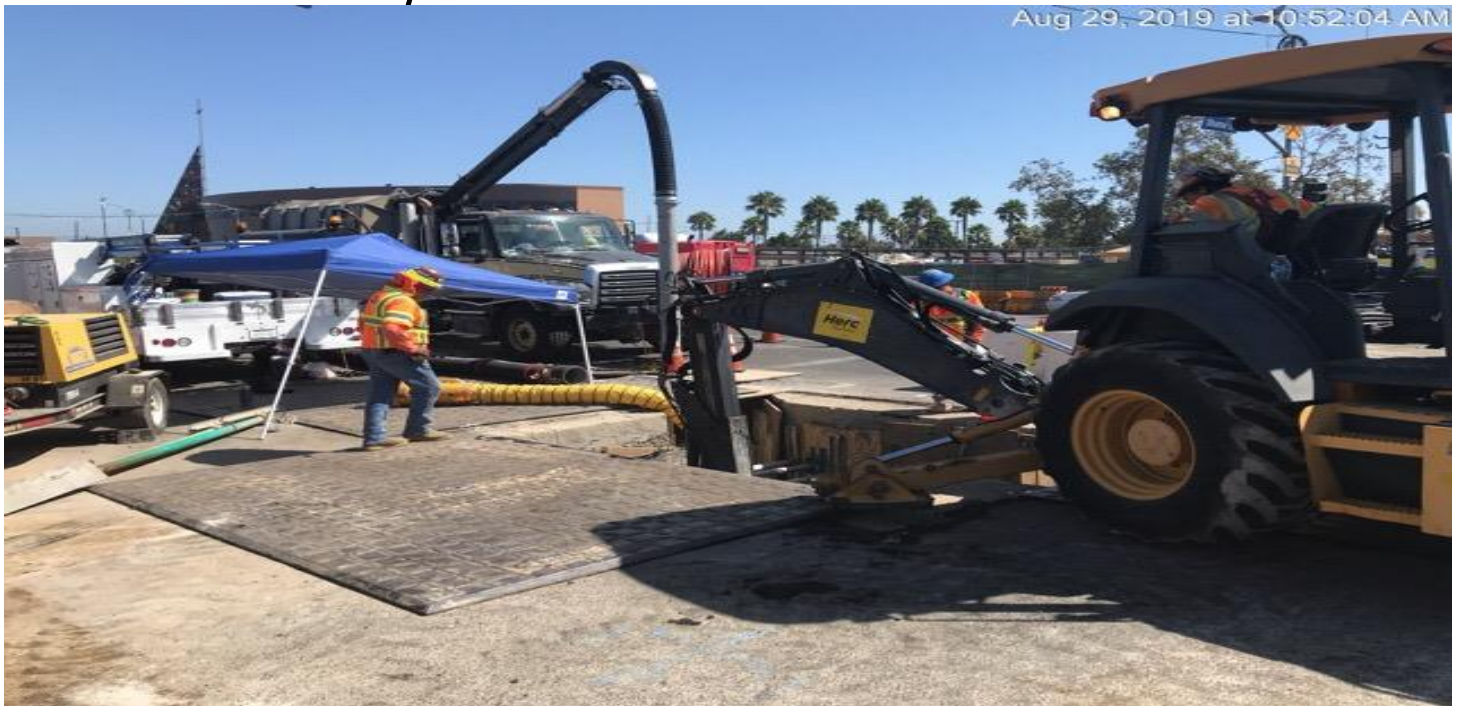
EXPOSITION/CRENSHAW STATION – Continued relocation of sewer manhole on N/W corner of Obama and Crenshaw Blvd.
