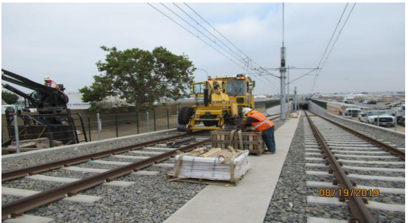
UG1- HCC at south portal of UG1 transferring material boxes using speed swing.
