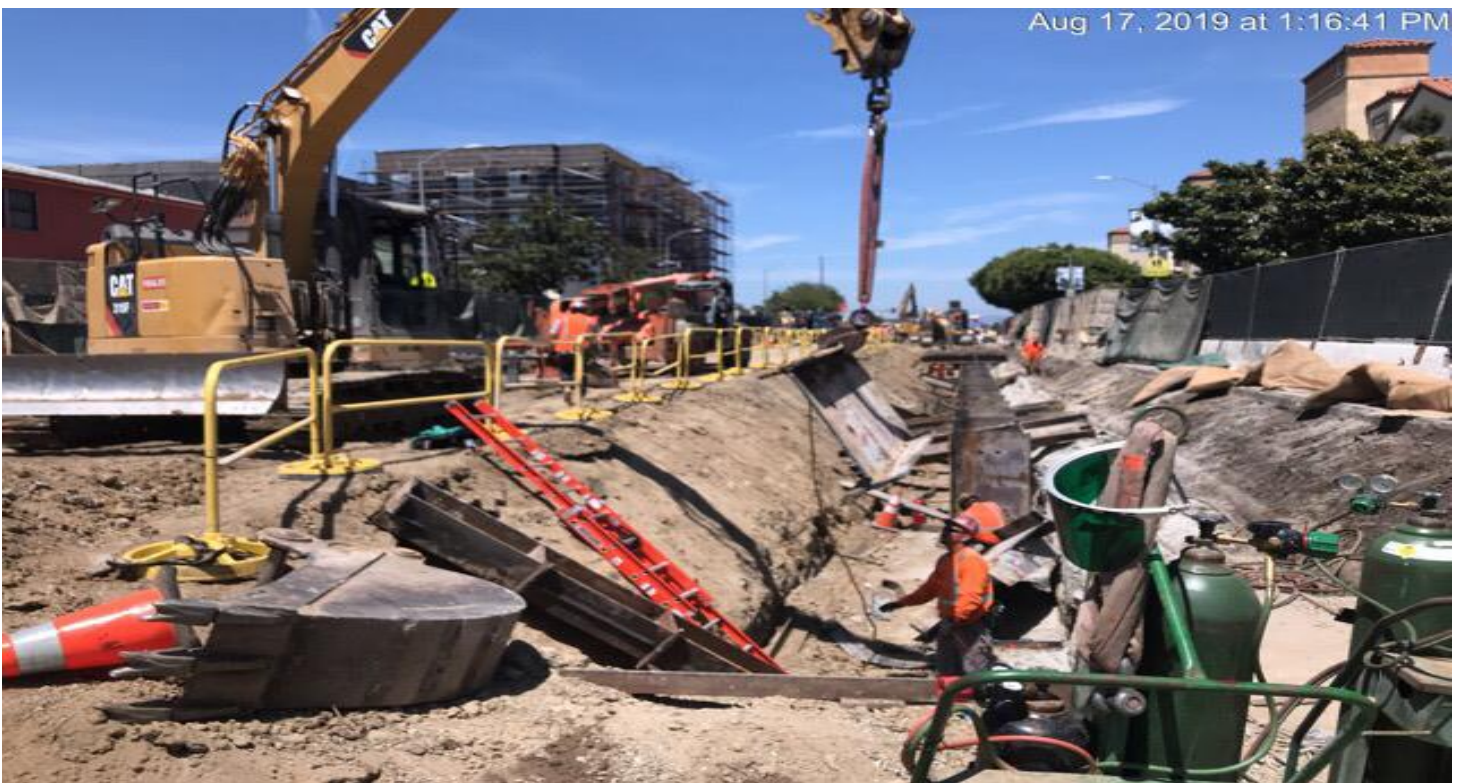
UG3- Continued removal of beams and northbound/southbound piles at 63rd and Crenshaw Blvd.
