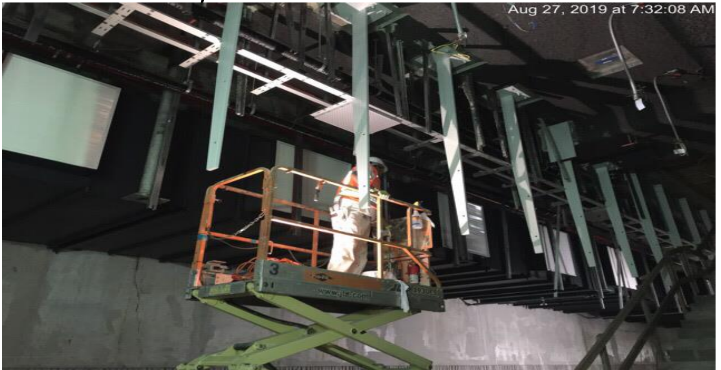
LEIMERT PARK STATION- Continued painting of northbound OTE vent duct at the invert level.
