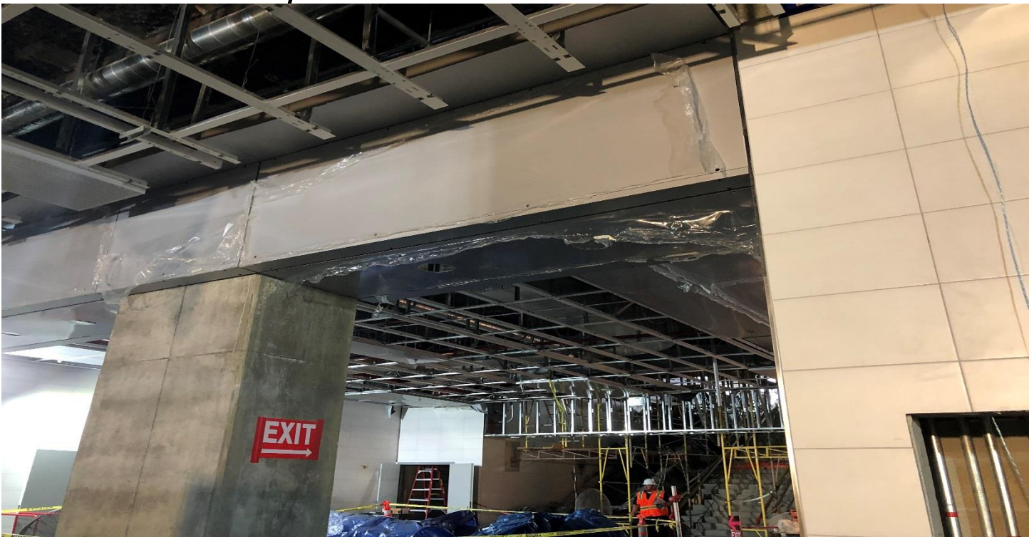
LEIMERT PARK STATION- Installation of overhead directional panels above the paid area of the concourse level.
