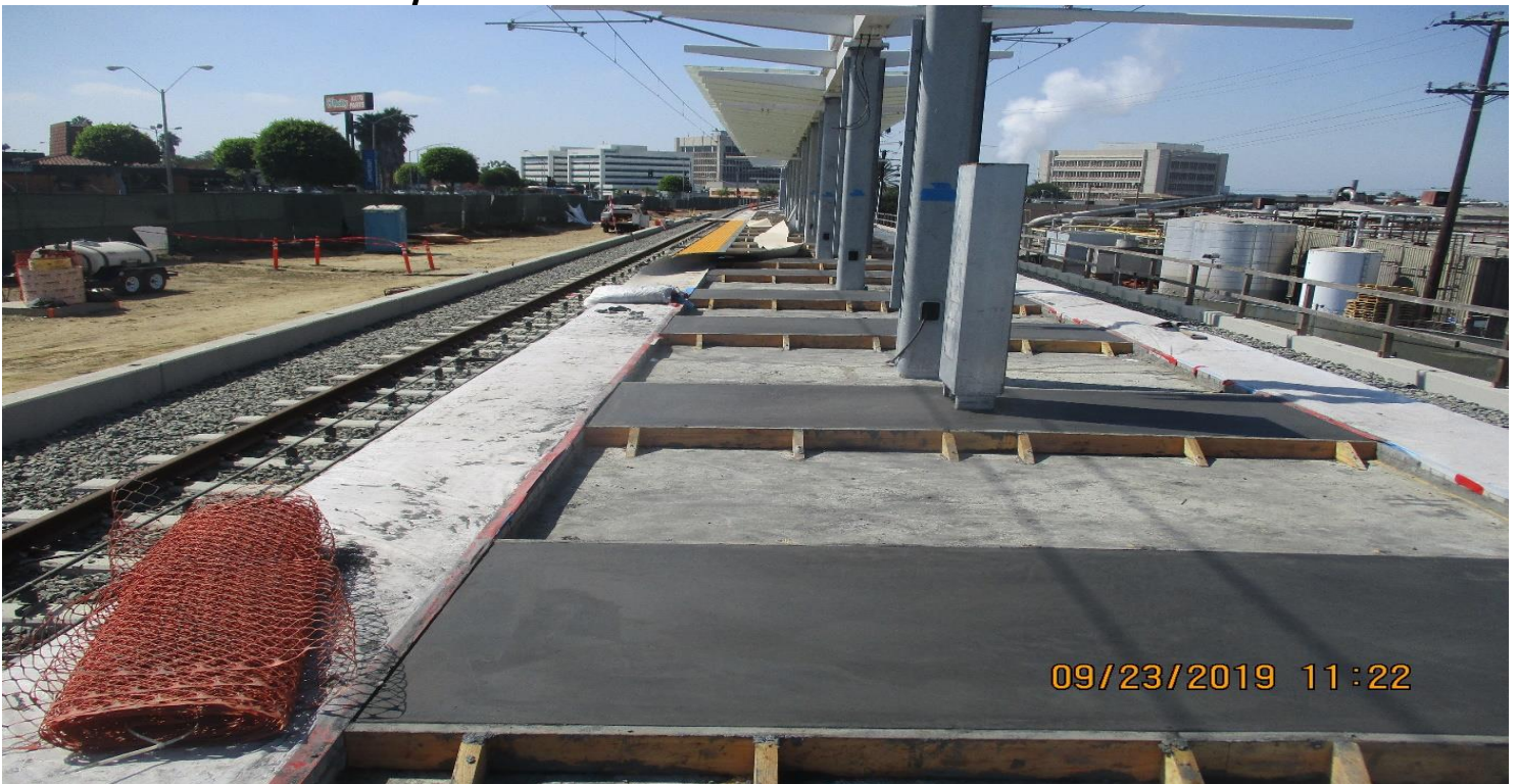
DOWNTOWN INGLEWOOD STATION- E Z Contracting Placing concrete floor on platform at La Brea Station.
