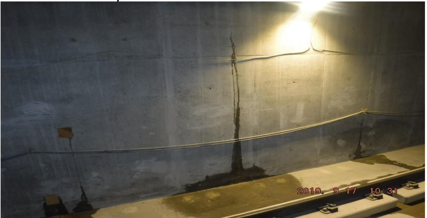
UG3- UG3- STA285+00 Looking North- Water infiltration.
