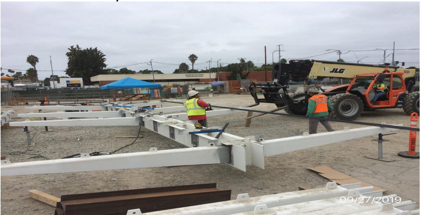
EXPOSITION/CRENSHAW STATION – Preparing canopy cantilever joints and outrigger fit up at the plaza level.
