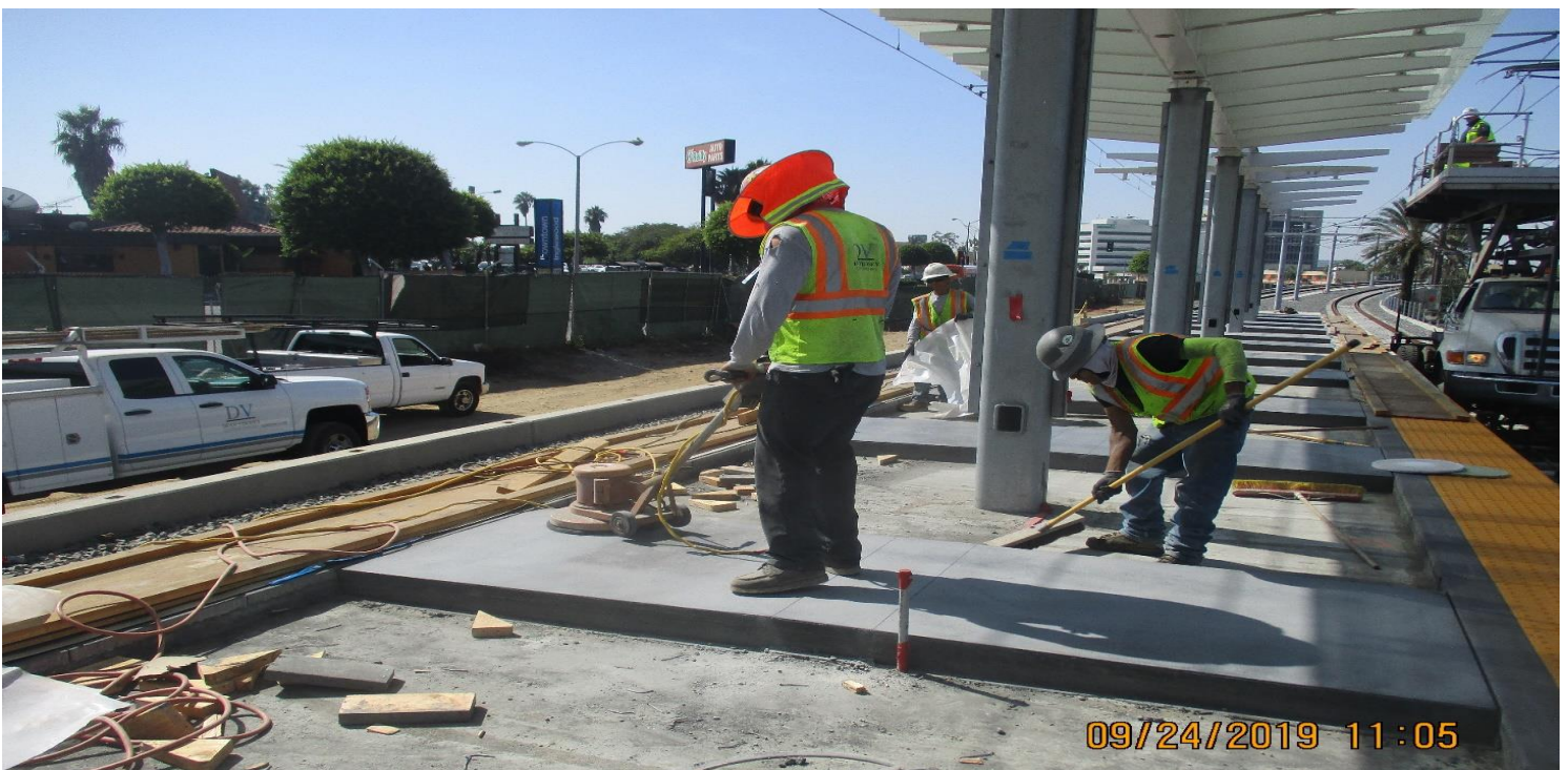
DOWNTOWN INGLEWOOD STATION- DV Contracting Stripping forms on concrete floor on platform at La Brea Station.
