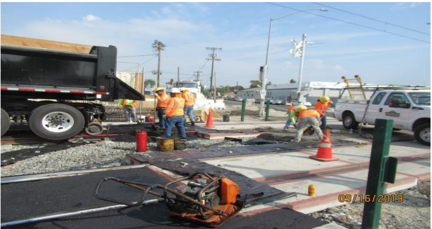
FLORENCE/HINDRY - WSCC placing Asphalt on SB track at Hindry grade crossing south side.
