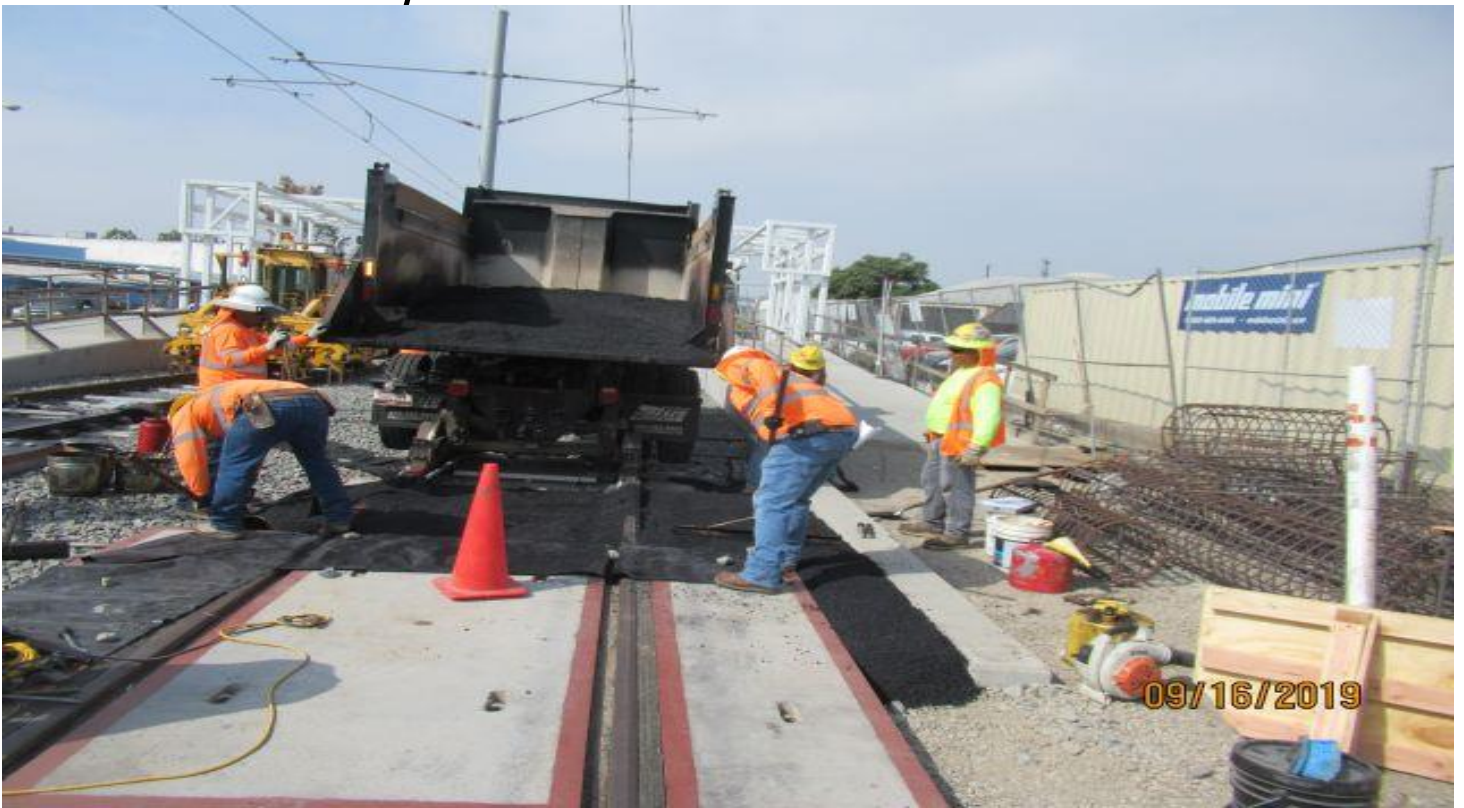
FLORENCE/HINDRY - WSCC AC area at Hindry grade crossing SB track.
