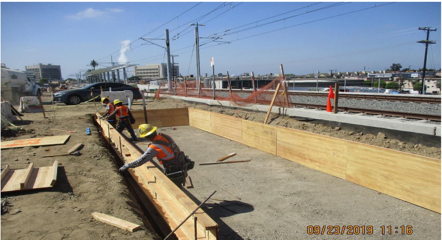
DOWNTOWN INGLEWOOD STATION- WSCC Forming for bath room building foundation at La Brea Station.
