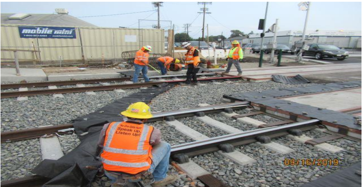
FLORENCE/HINDRY - WSCC AC crew along with QC inspector going over asphalt install plan at Hindry grade crossing south side.
