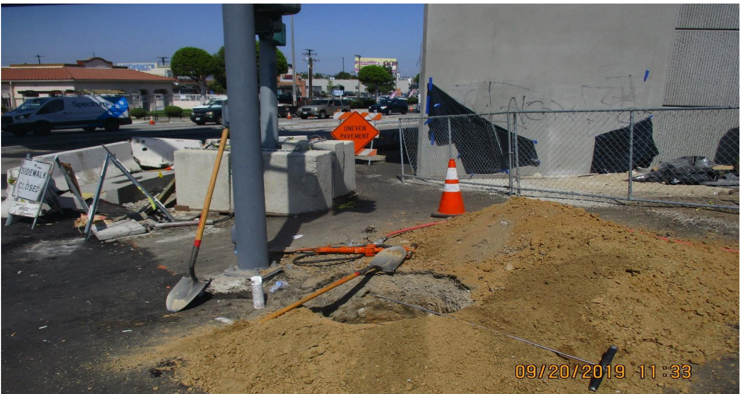
FLORENCE/LABREA STREET - Select Electric Pot hole for TS pole foundation at NWC of La Brea and Florence.
