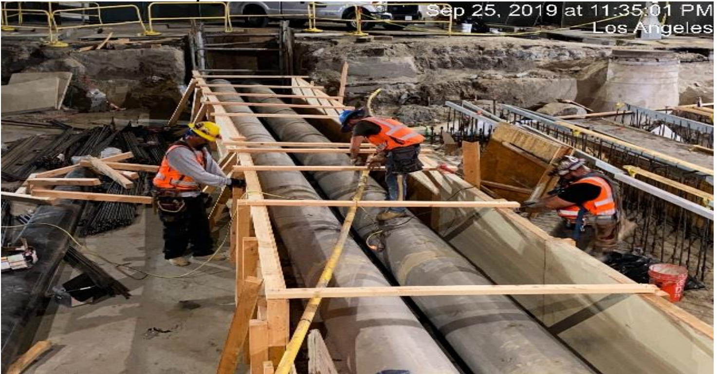
UG3- Installation of A – Line reinforced concrete pipe storm drain on the intersection of 67th St and Crenshaw Blvd.
