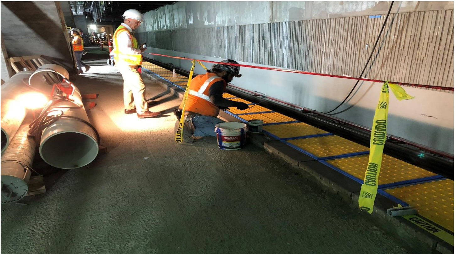
LEIMERT PARK STATION- Continued installation of edge pavers on the north and south bound platform level.
