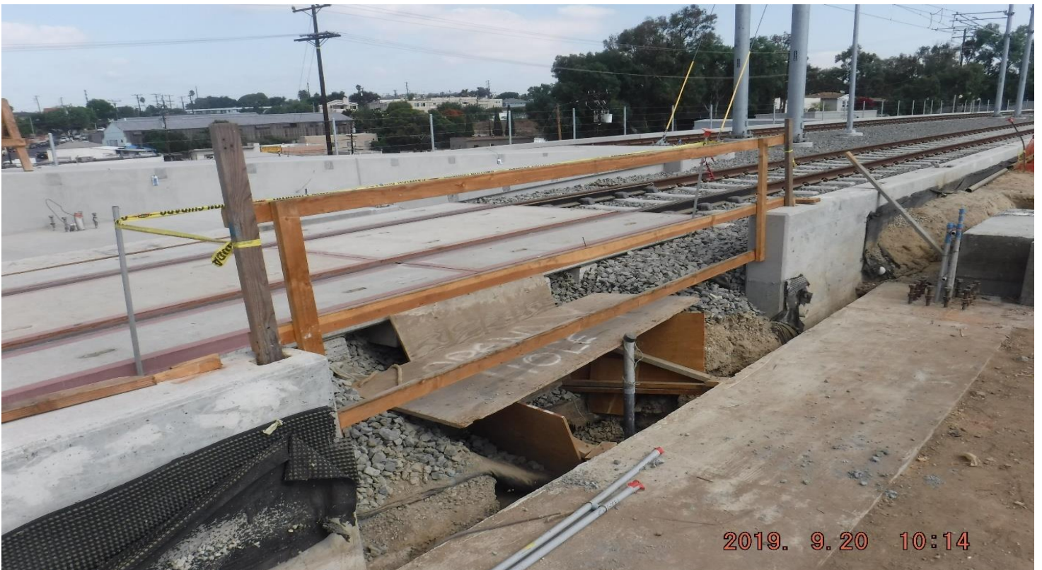
FLORENCE/LABREA STREET - Looking North- Disturbed track structure.
