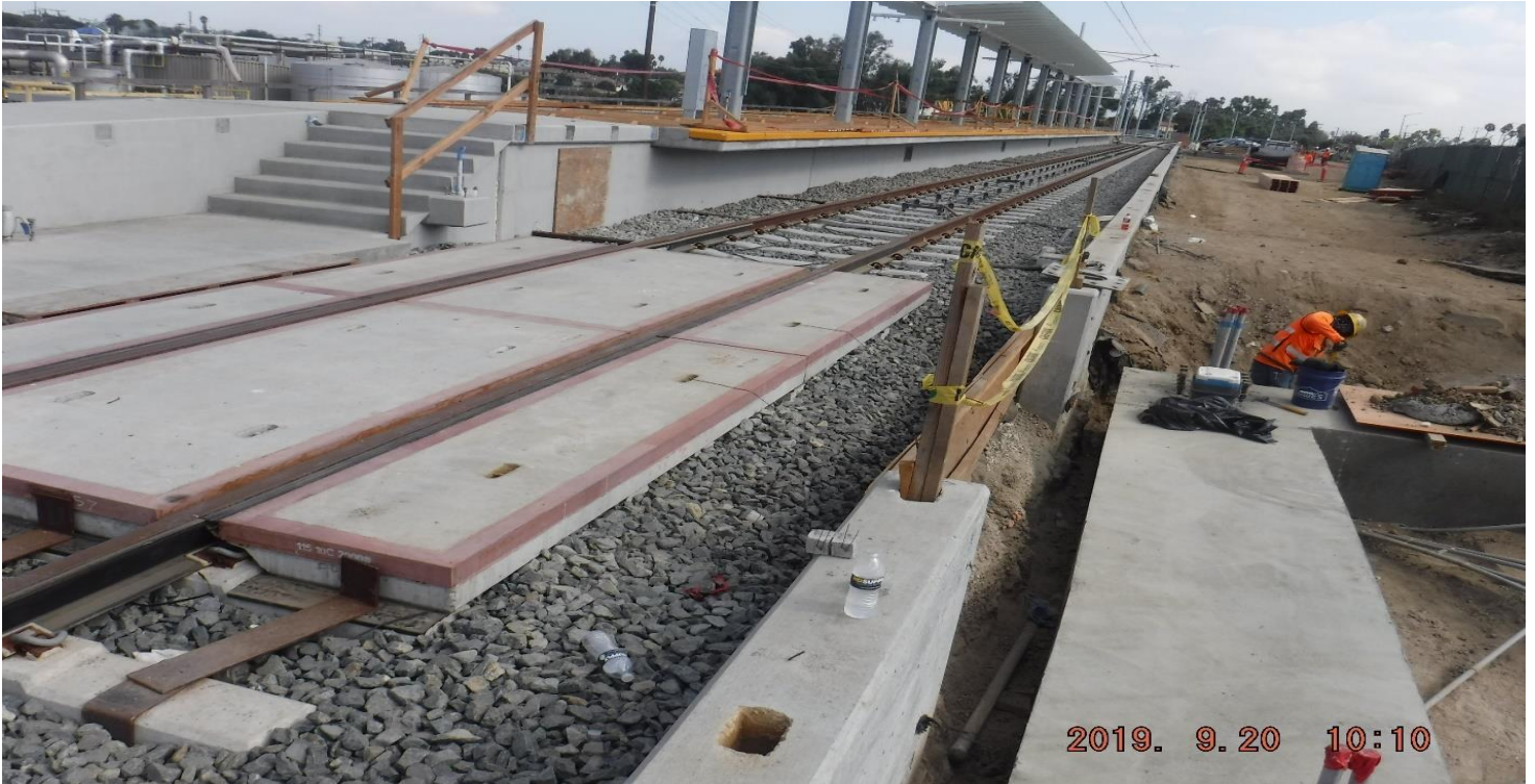
FLORENCE/LABREA STREET - Looking North- Disturbed track structure.
