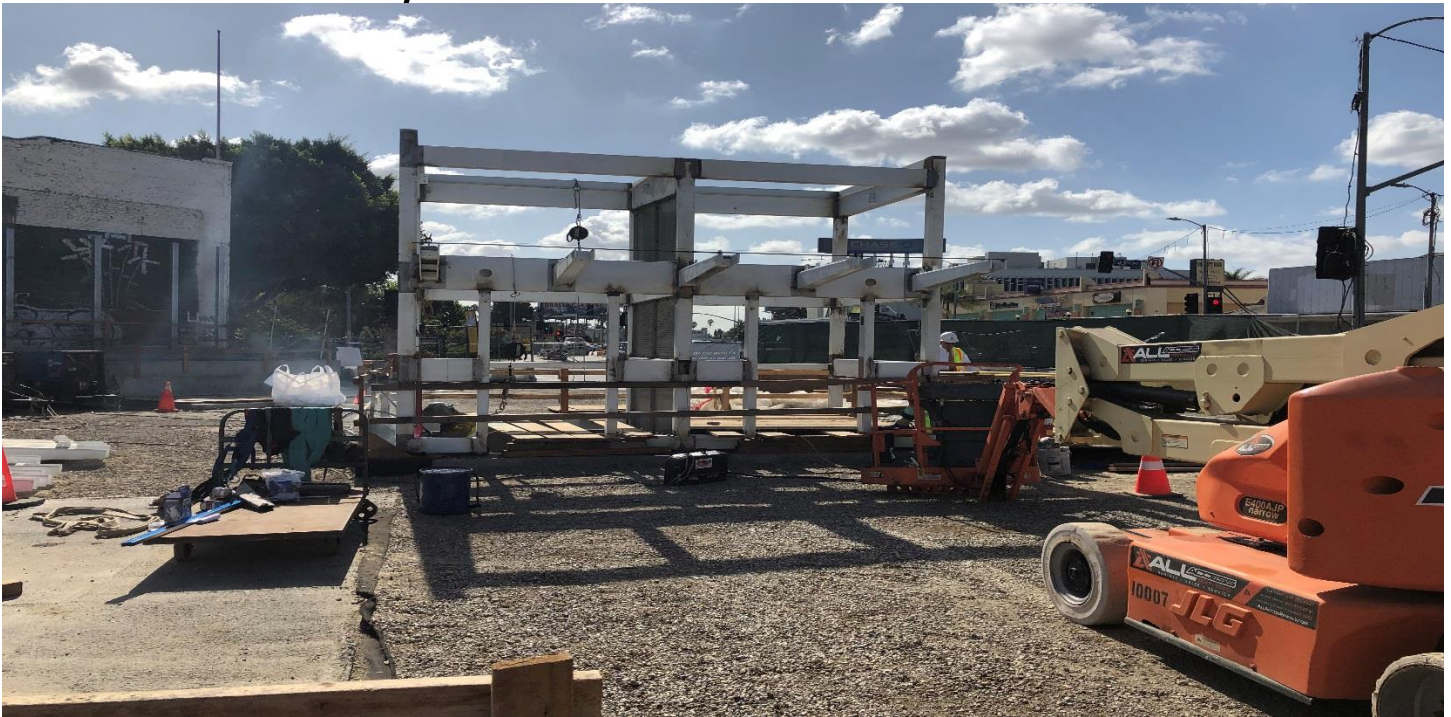
LEIMERT PARK STATION- Continued installation of entrance canopy steel for Elevators 1 & 2 at the plaza level.
