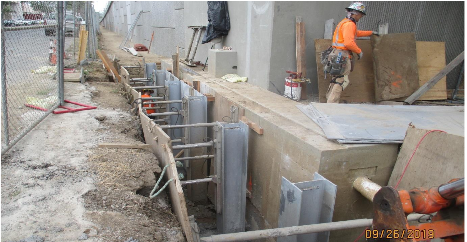
405 BRIDGE - Removal of the temporary shoring for the COS protection at abutment 5 of the 405 bridge.
