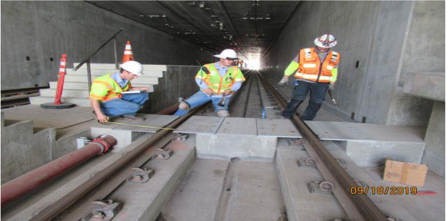
UG1- Metro & WSCC measuring flangeway gaps on walkway plates in UG1.
