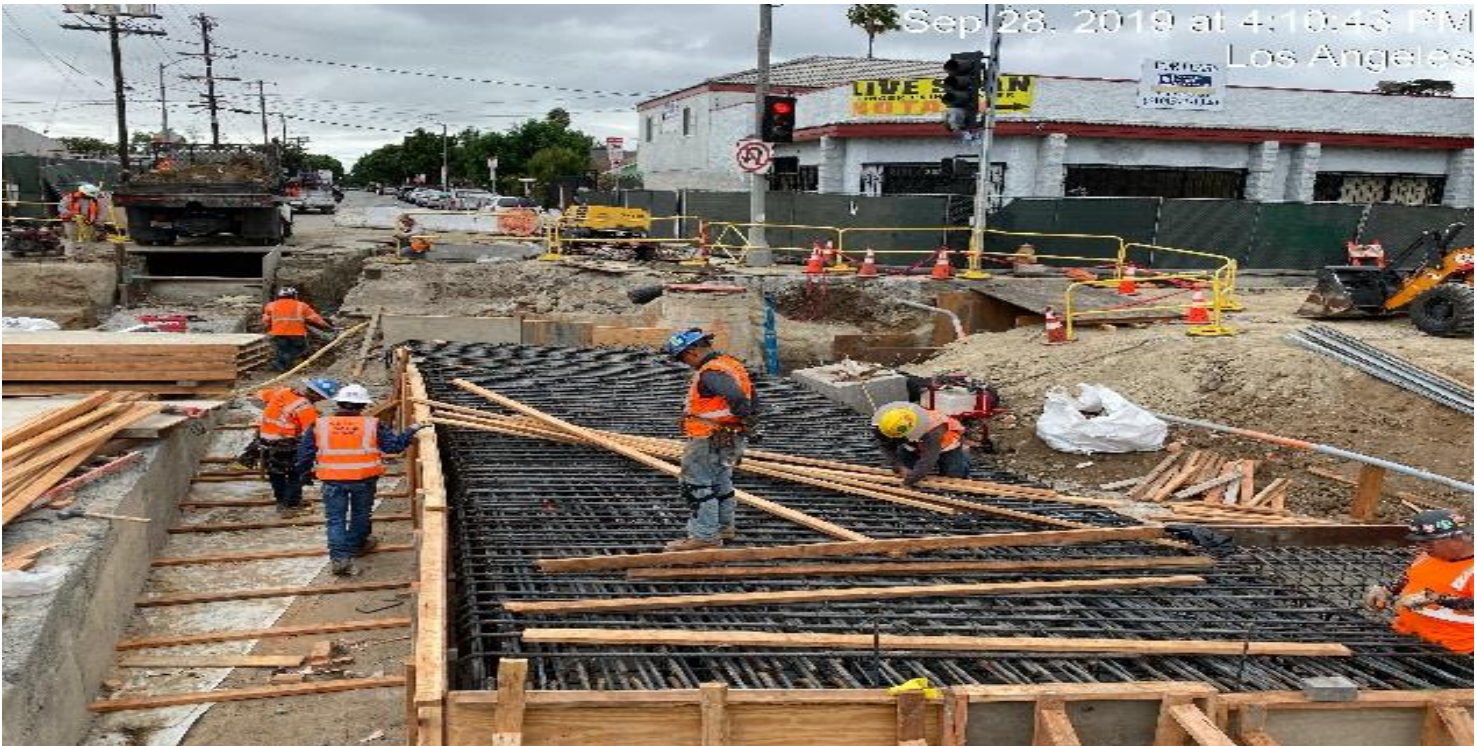
UG3- Installation of steel bars for LADWP duct bank on the southwest of 67th St & Crenshaw Blvd.
