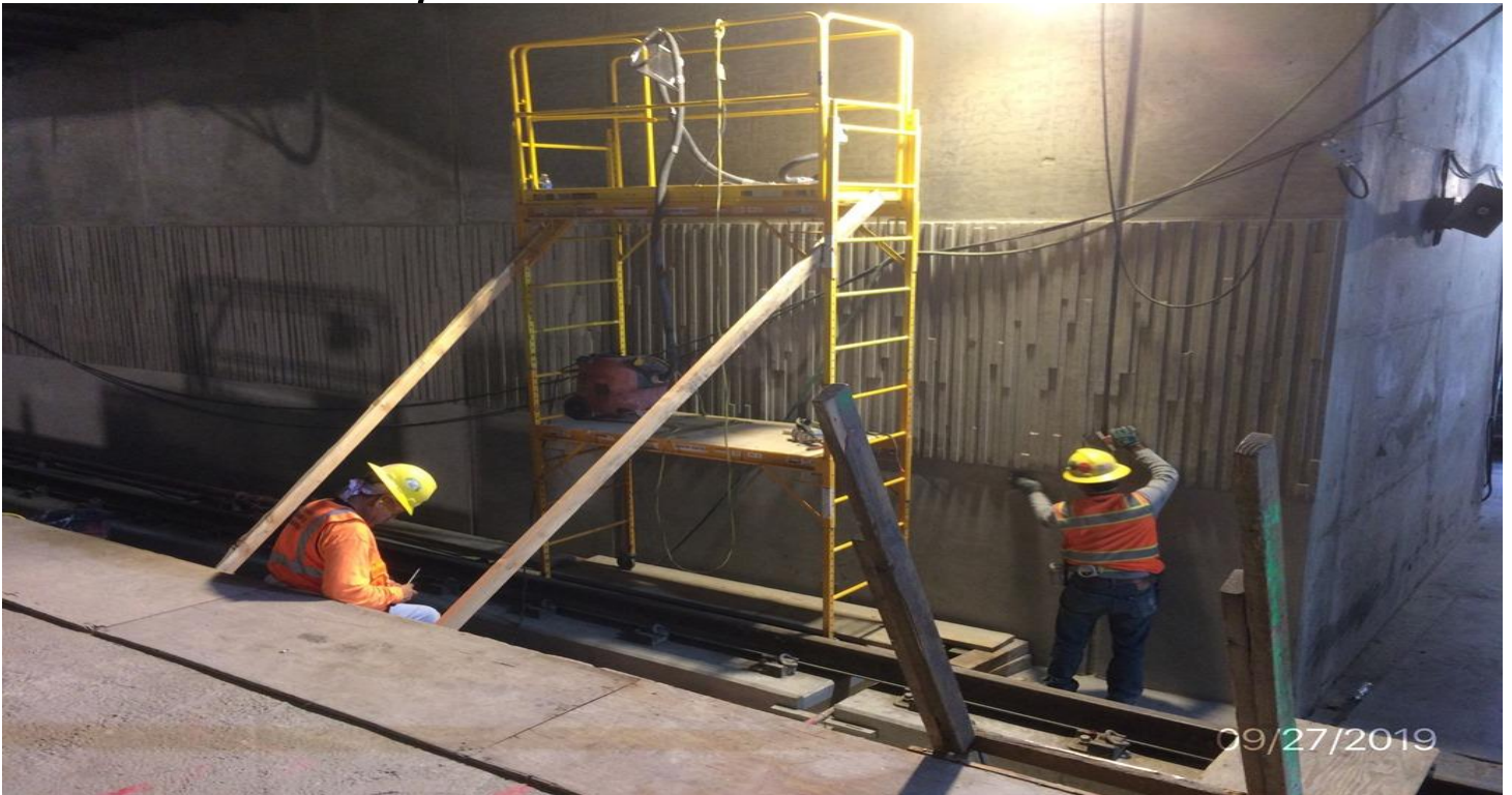
EXPOSITION/CRENSHAW STATION – Continued finish work of the concrete wall on the east side of Track 4 at the platform level.
