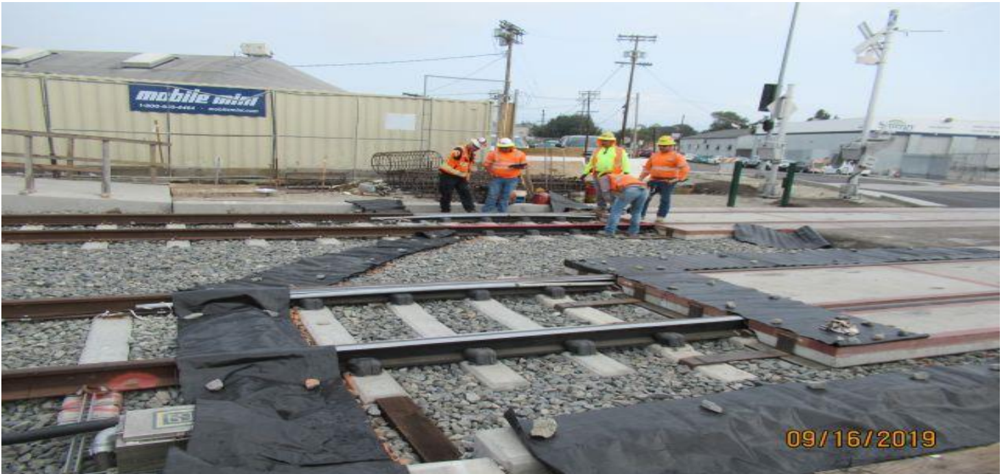
FLORENCE/HINDRY - WSCC AC crew laying out asphalt install on south side of xing at Hindry.
