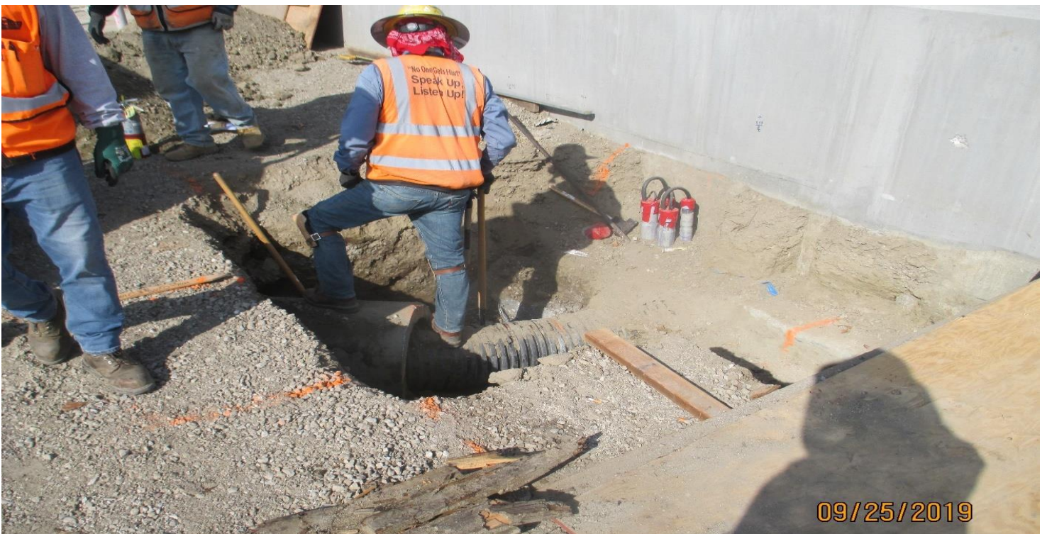
FLORENCE/HINDRY - Storm drain line connection to be made just west of the Hindry Station.
