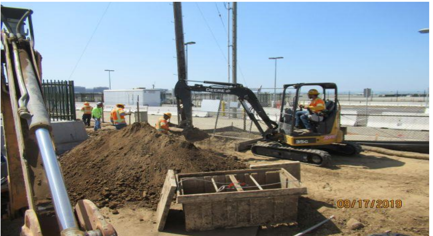
111 TH STREET- WA Rasic using mini ex. to excavate & relocate hand hold.
