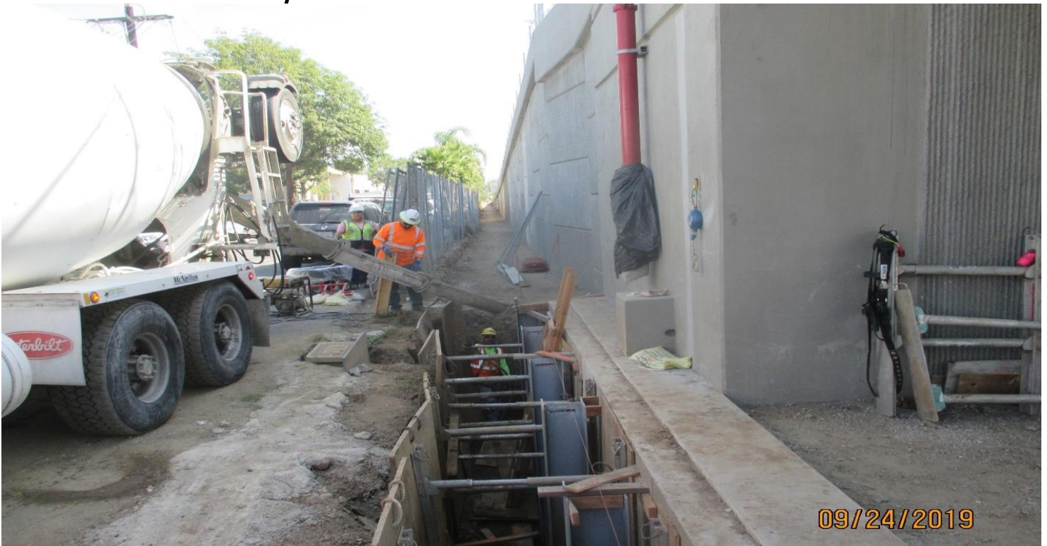
405 BRIDGE - Placing concrete to set the I beam shoring for the COS protection at the 405 bridge.
