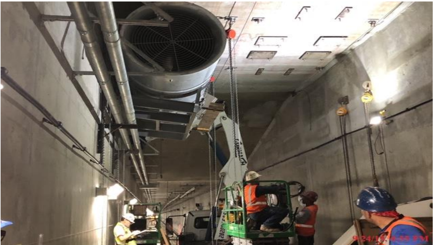
UG3- Continued installation of tunnel booster fans at station 307+40 in the southbound tunnel.
