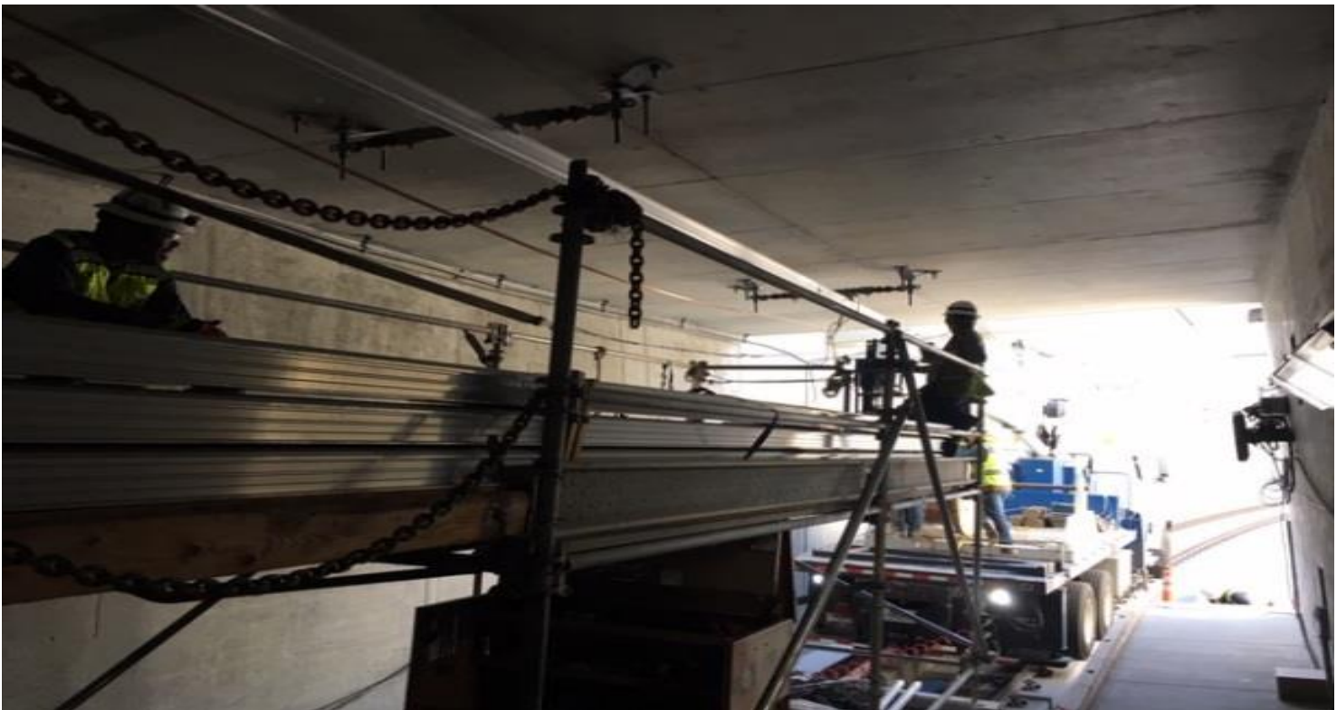
UG3- Continued installation of overhead conductor rail supports at the southbound portal.
