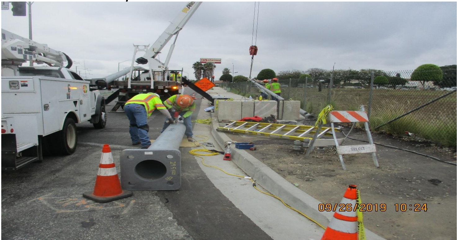
FLORENCE/LA BREA- Select Electric Stand TS and SL pole on N EC of La Brea and Florence.
