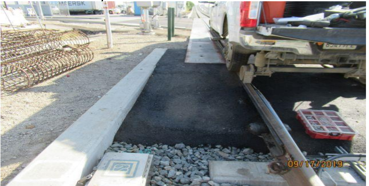
FLORENCE/HINDRY - SB track at Hindry grade crossing newly placed AC for Ped. walkway access.
