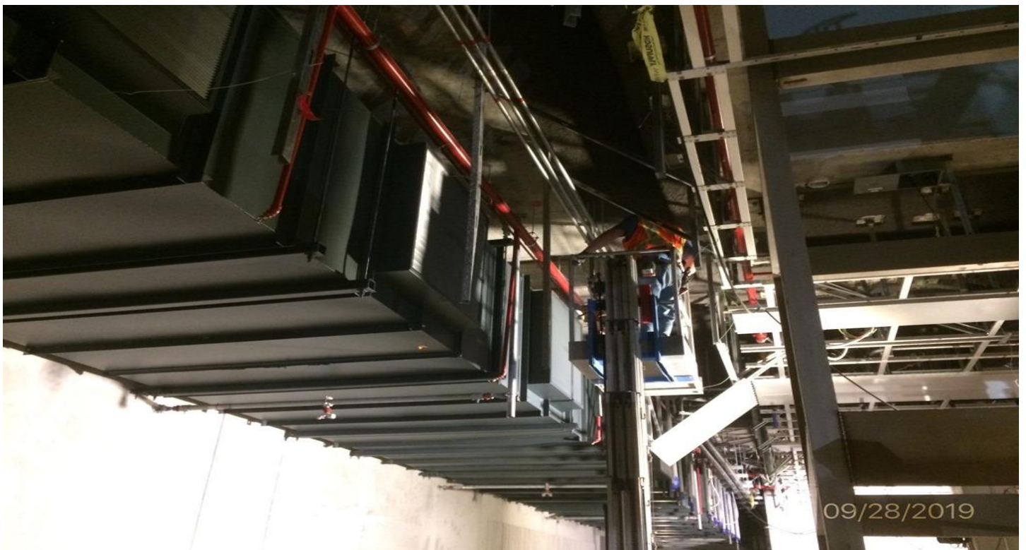
MARTIN LUTHER KING JR. STATION- Installation of overhead fire alarm conduit at the platform level.
