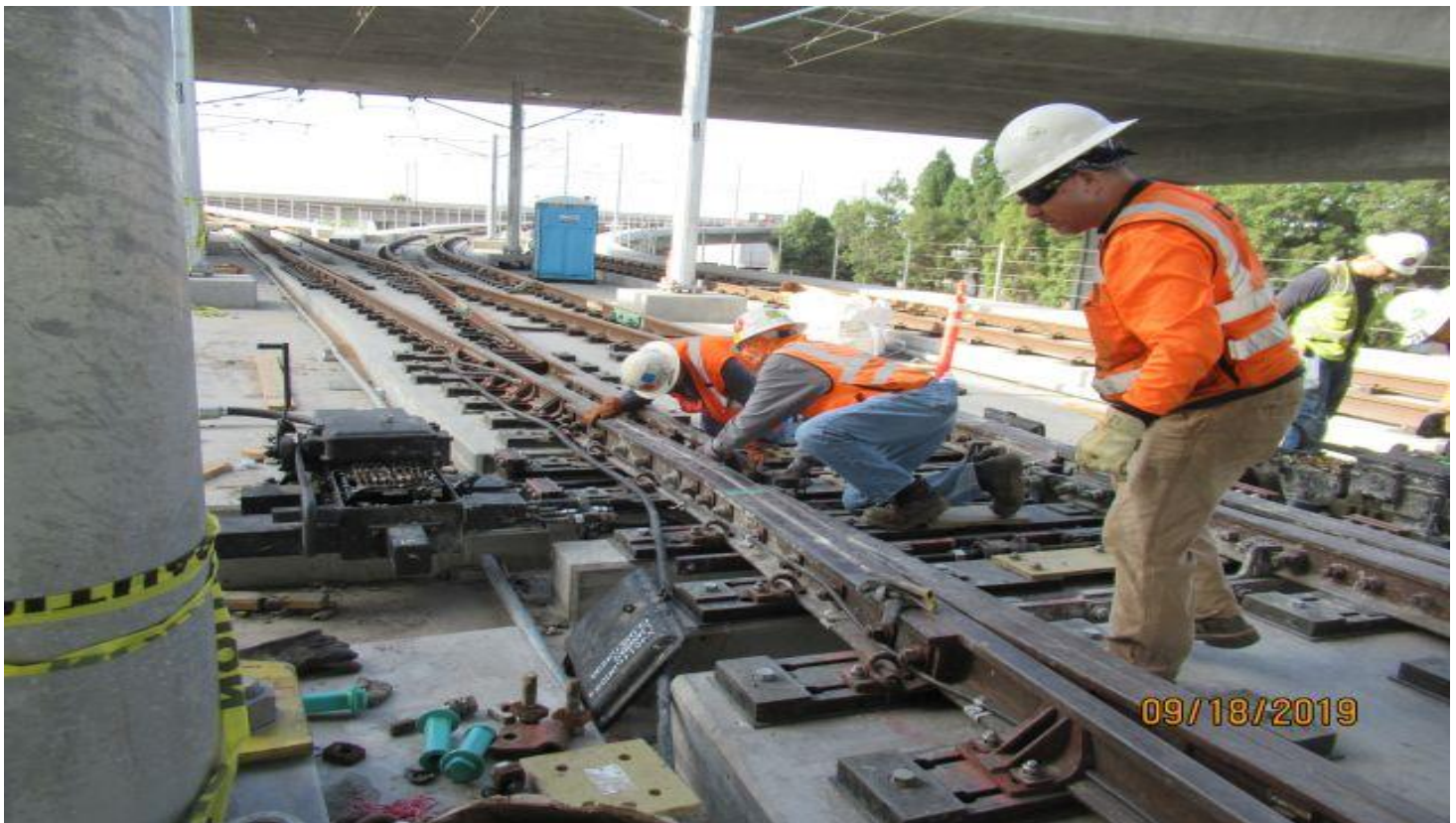
GREENLINE WYE- HCC adjusting gauge on Movable Point Frog.
