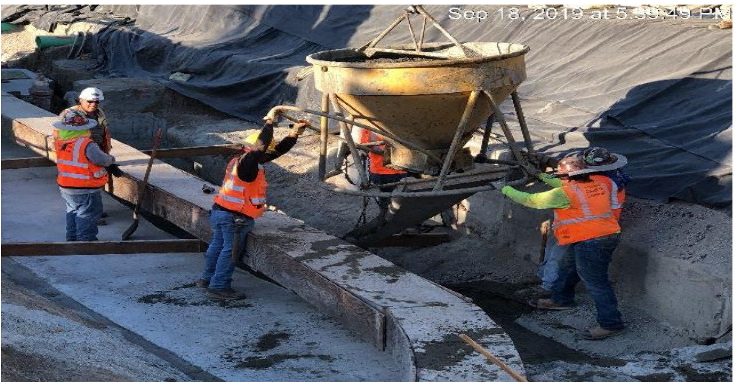
MARTIN LUTHER KING JR. STATION- Slurry installation for C – Line reinforced concrete box storm drain at the topside.
