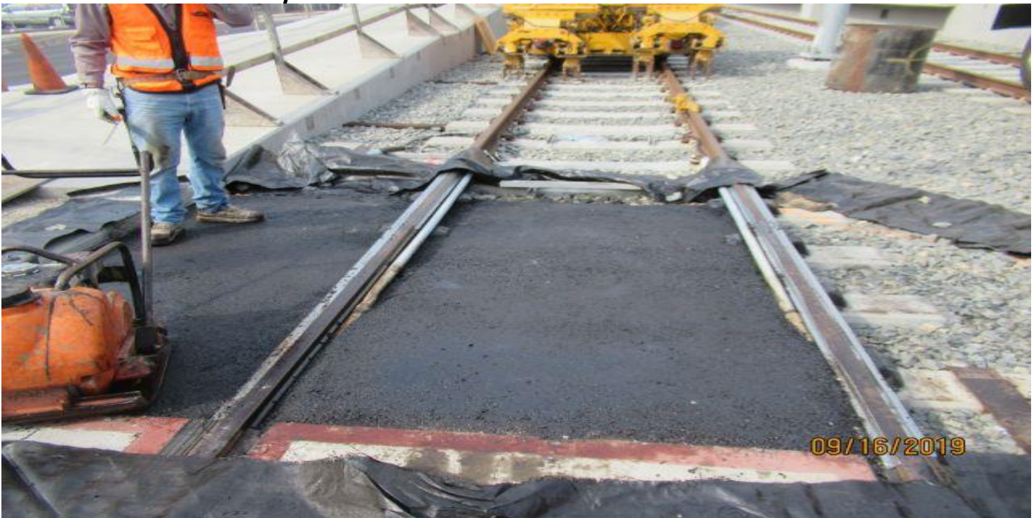
FLORENCE/HINDRY - NB track south side of Xing Hindry grade crossing with End restraint walkway ramp installed.
